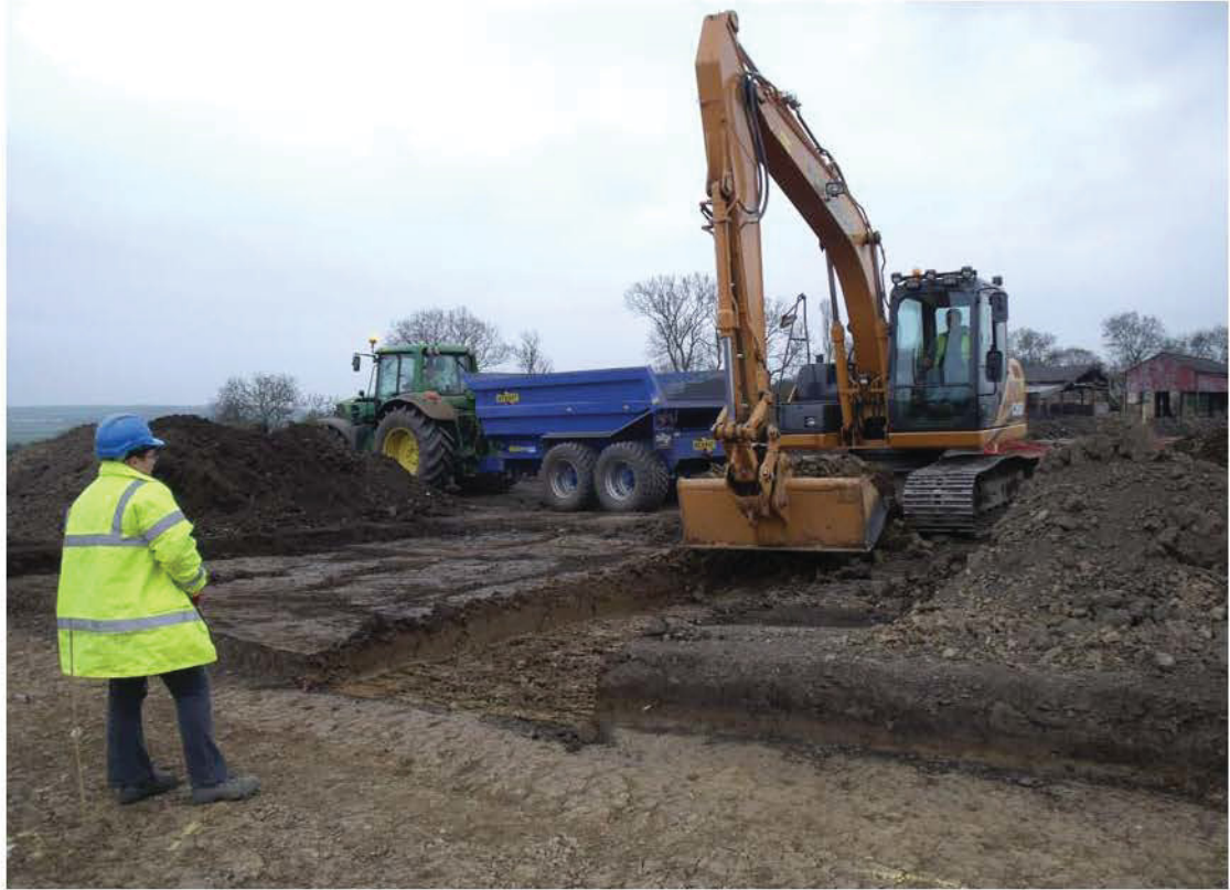
Plate 9: Working shot, machine clearance of overburden for Area A extension, looking south
