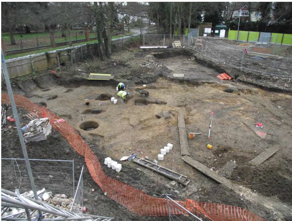
Plate 1: Area of excavation facing southeast The irregular shape of the trench is abundantly apparent in this shot
