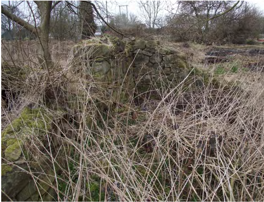
Plate 15. View of partition wall in derelict buildings, looking NNW
