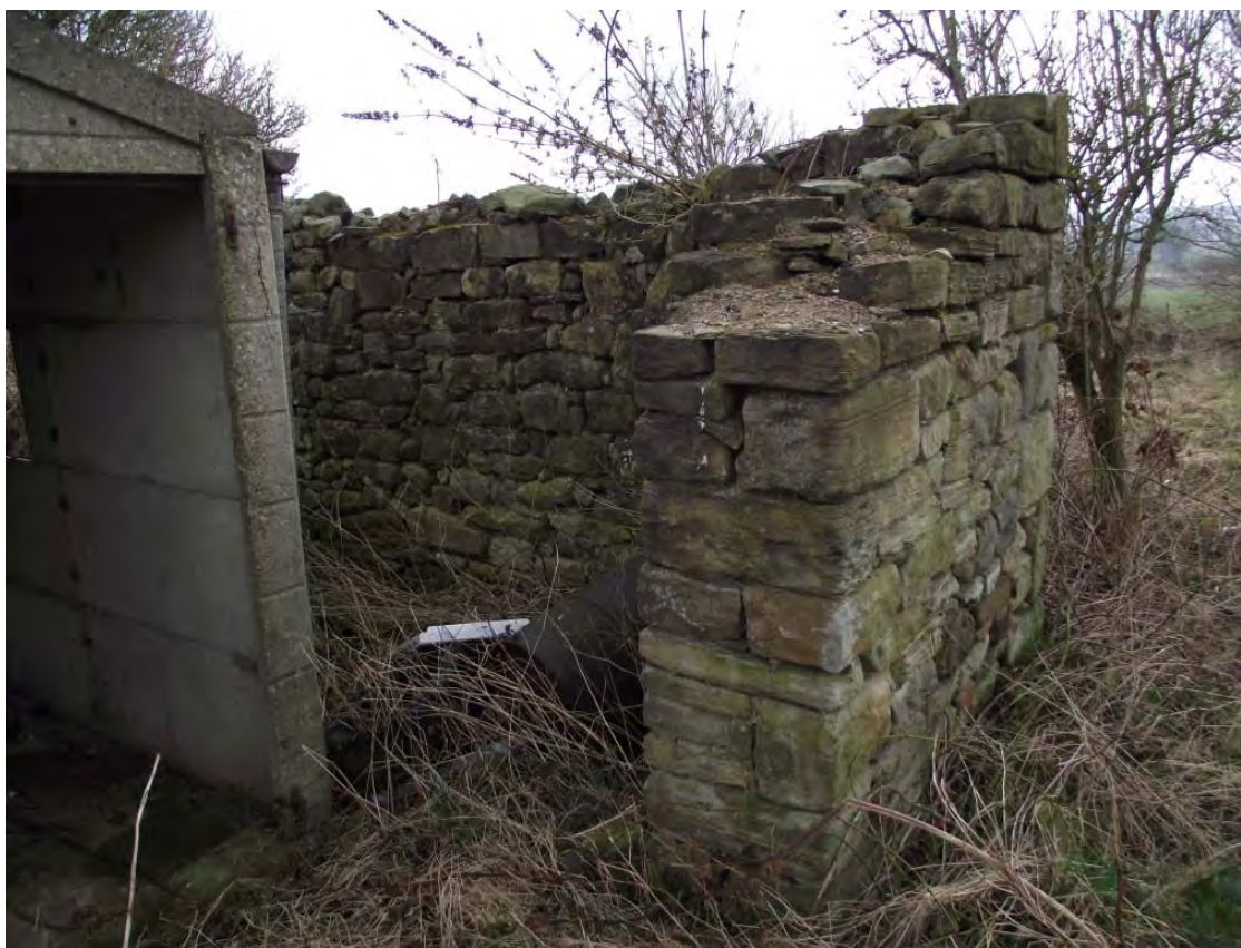
Plate 14. Detail of western entrance to derelict buildings, looking south-east
