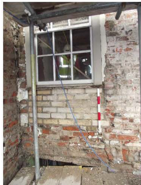
Plate 29: West-facing (rear) elevation, southern element, brick infill below replacement window in first floor (0.5m scale)
