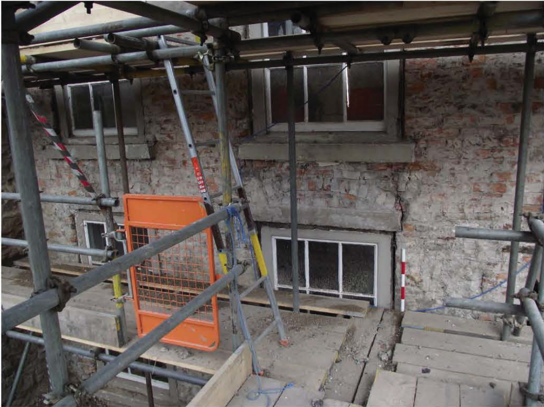
Plate 22: West-facing (rear) elevation, northern element, brickwork arches above ground floor windows (0.5m scale)
