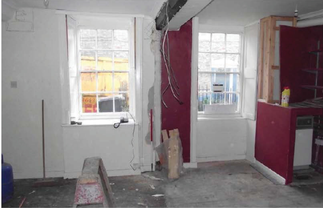
Plate 36: Front element, ground floor, study and flat lobby, partition wall removed (1m scale)
