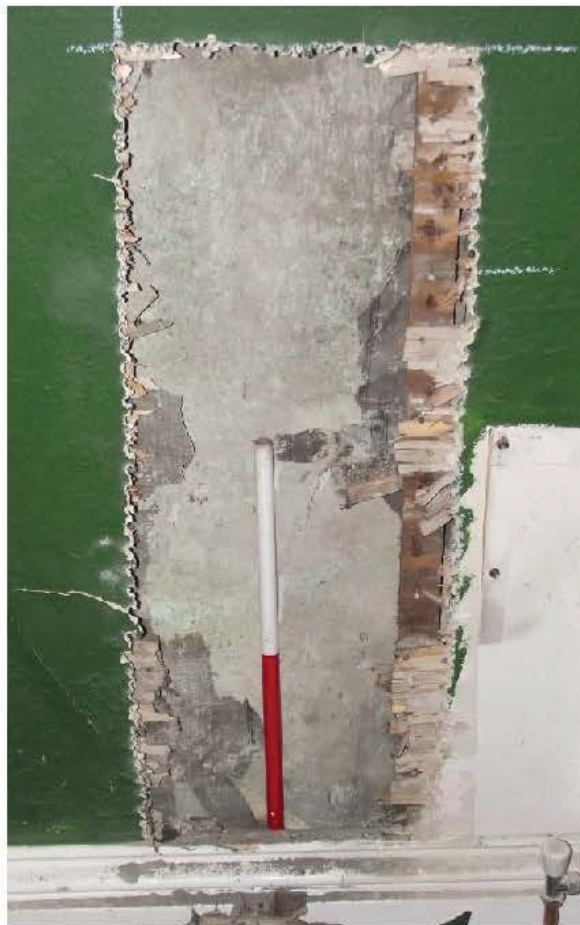
Plate 62: Northern rear element, first floor, Bedroom 1, service installation area in north wall (0.5m scale)
