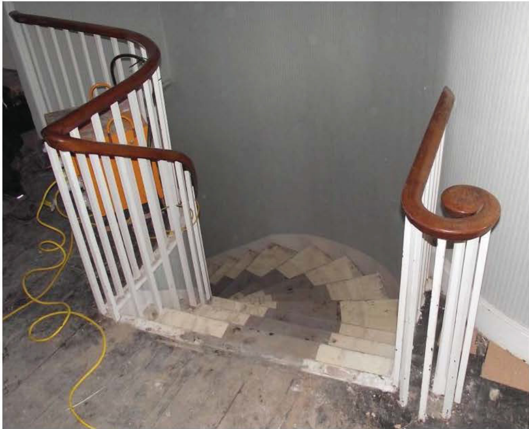
Plate 57: Southern rear element, main staircase, from first floor landing (view, no scale)
