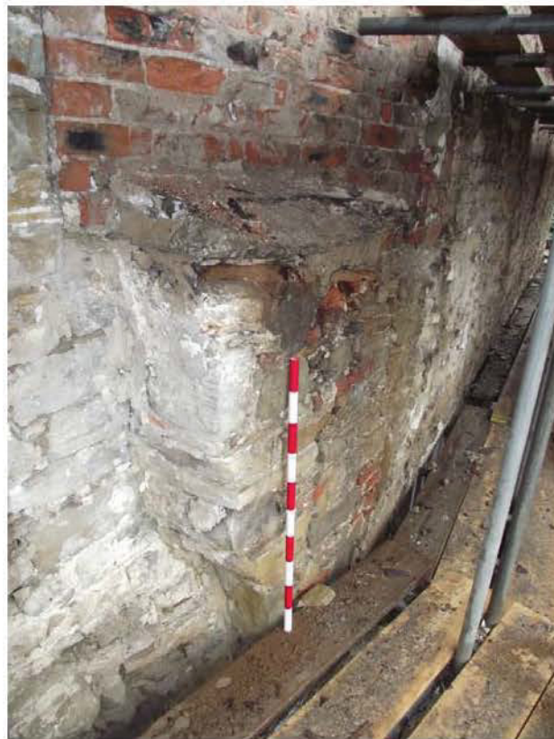
Plate 18: North-facing (side) elevation, front element, projecting masonry of capped chimney (1m scale)
