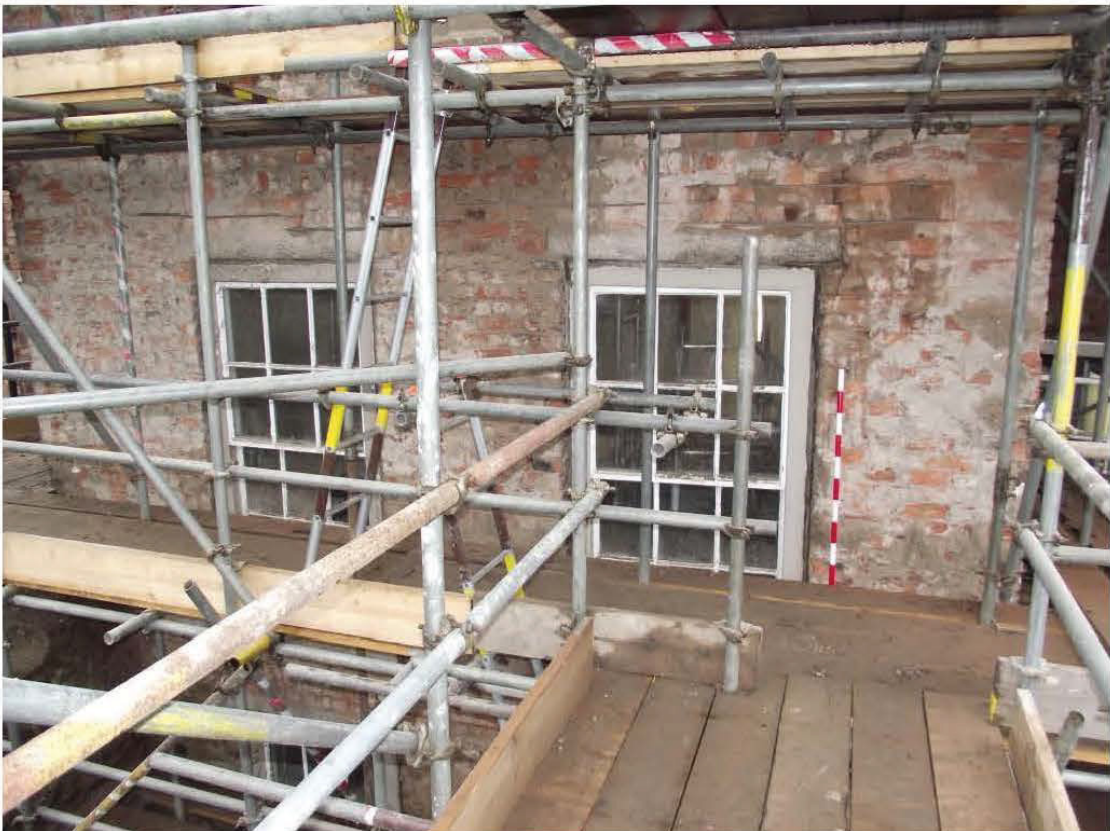
Plate 23: West-facing (rear) elevation, northern element, brickwork arches above first floor windows (1m scale)
