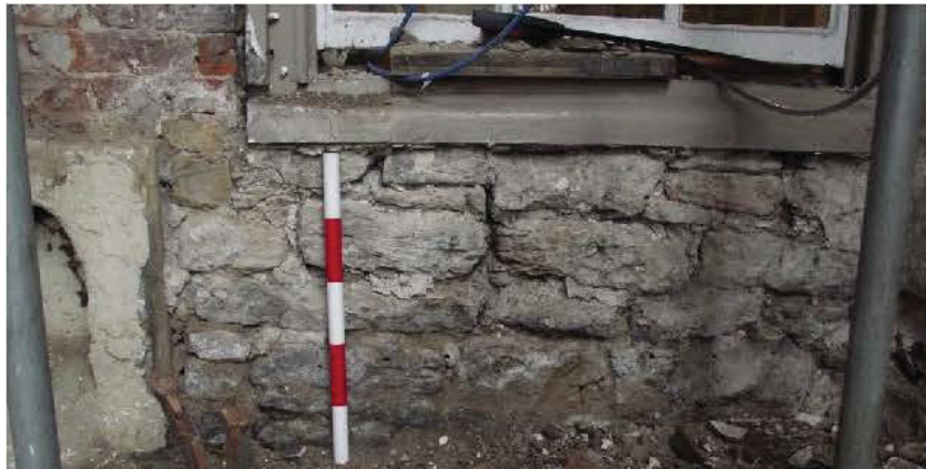
Plate 41: West-facing (rear) elevation, southern element, sandstone masonry below ground floor window (0.5m scale)
