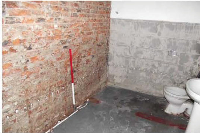
Plate 51: S-shaped rear extension, utility room/WC range, brickwork exposed in east wall (1m scale)
