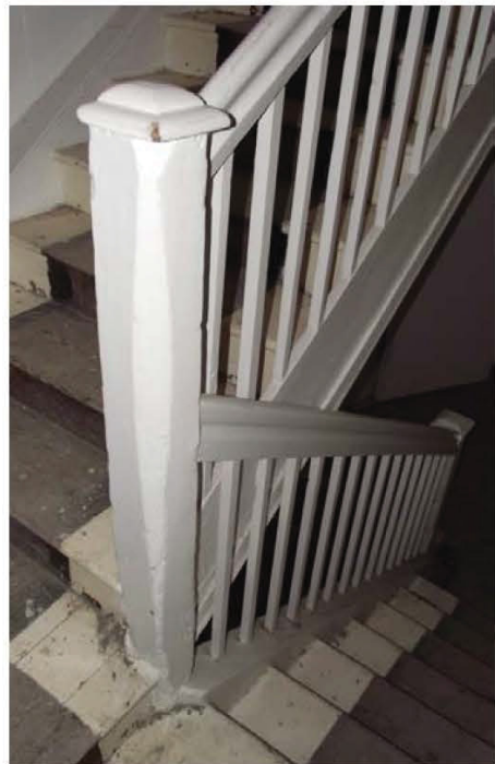
Plate 56: Northern rear element, staircase, balustrade at half-landing between first and second floor (view, no scale)
