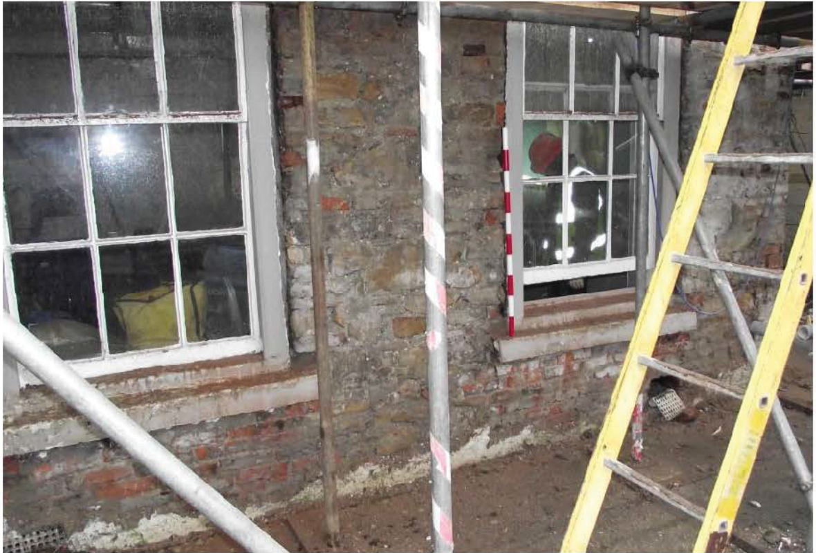
Plate 17: West-facing (rear) elevation, northern element, masonry with brick infill below windows (1m scale)
