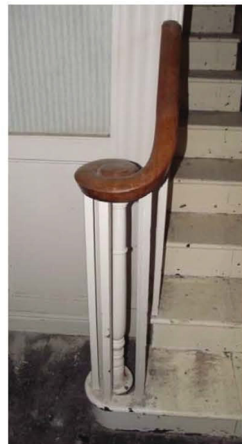
Plate 35: Front element, ground floor, staircase from main lobby, balustrade detail (view, no scale)
