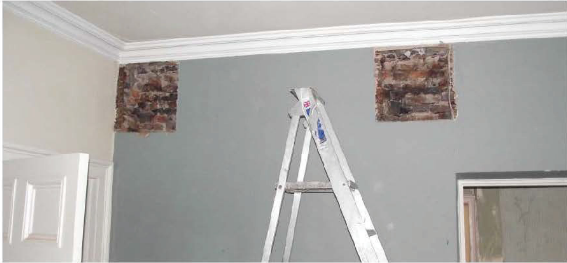
Plate 45: Northern rear element, ground floor, Reception Room 1, enabling holes in south wall (view, no scale)
