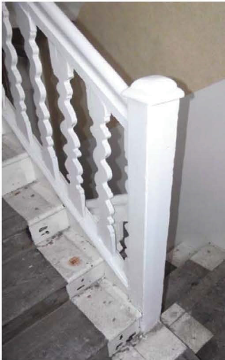
Plate 55: Northern rear element, staircase, balustrade at half-landing between ground and first floor (view, no scale)
