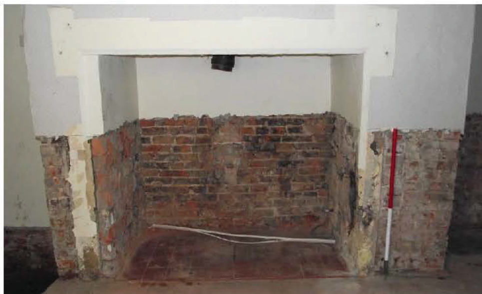
Plate 42: Southern rear element, ground floor, Reception Room 2, exposed masonry in fireplace (1m scale)
