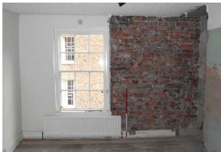
Plate 75: Front element, second floor, kitchen, exposed brickwork in east wall (1m scale)
