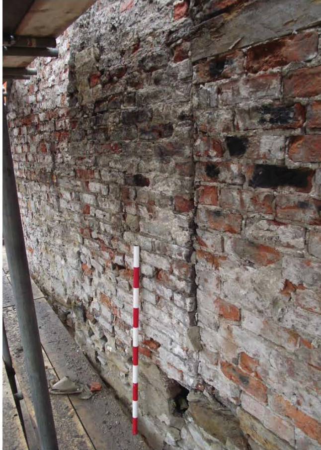
Plate 24: North-facing (side) elevation, front element, chimney breast (brickwork above sandstone masonry) (1m scale)
