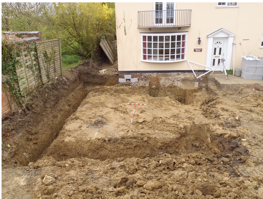
Plate 3, General view of excavated foundations, at the front of the property facing south (Scales 2m and 1m)
