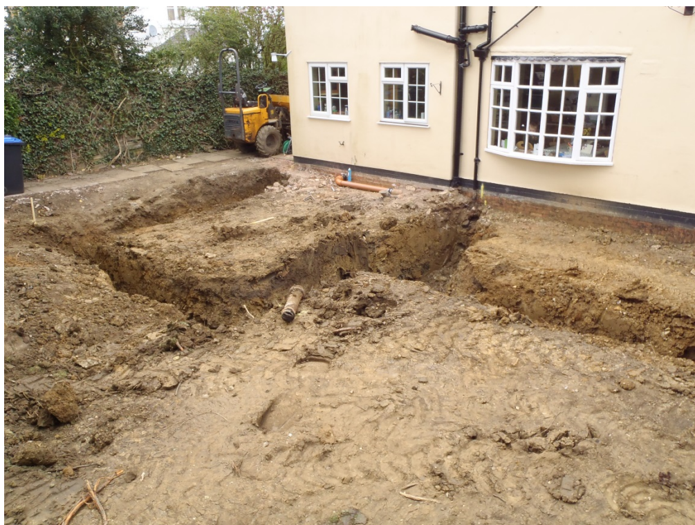
Plate 5, General view of excavated foundations, at the rear of the property facing northwest
