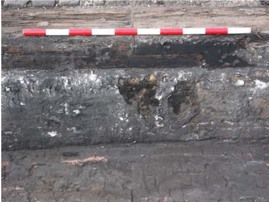
Plate 5-5 1841 Engine Shed, detail of inspection pit [1005] with L-shaped tenon joint in waybeam, looking north (scale 1m)
