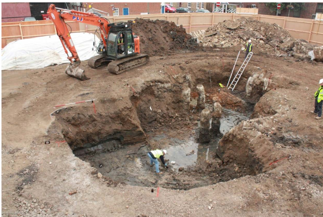
Plate 1 D1/18. Overall view of the excavation looking NE. Original 5m 2 trench in centre (with old piles) with later extensions to trench to the NW and SE. Scale 2m.
