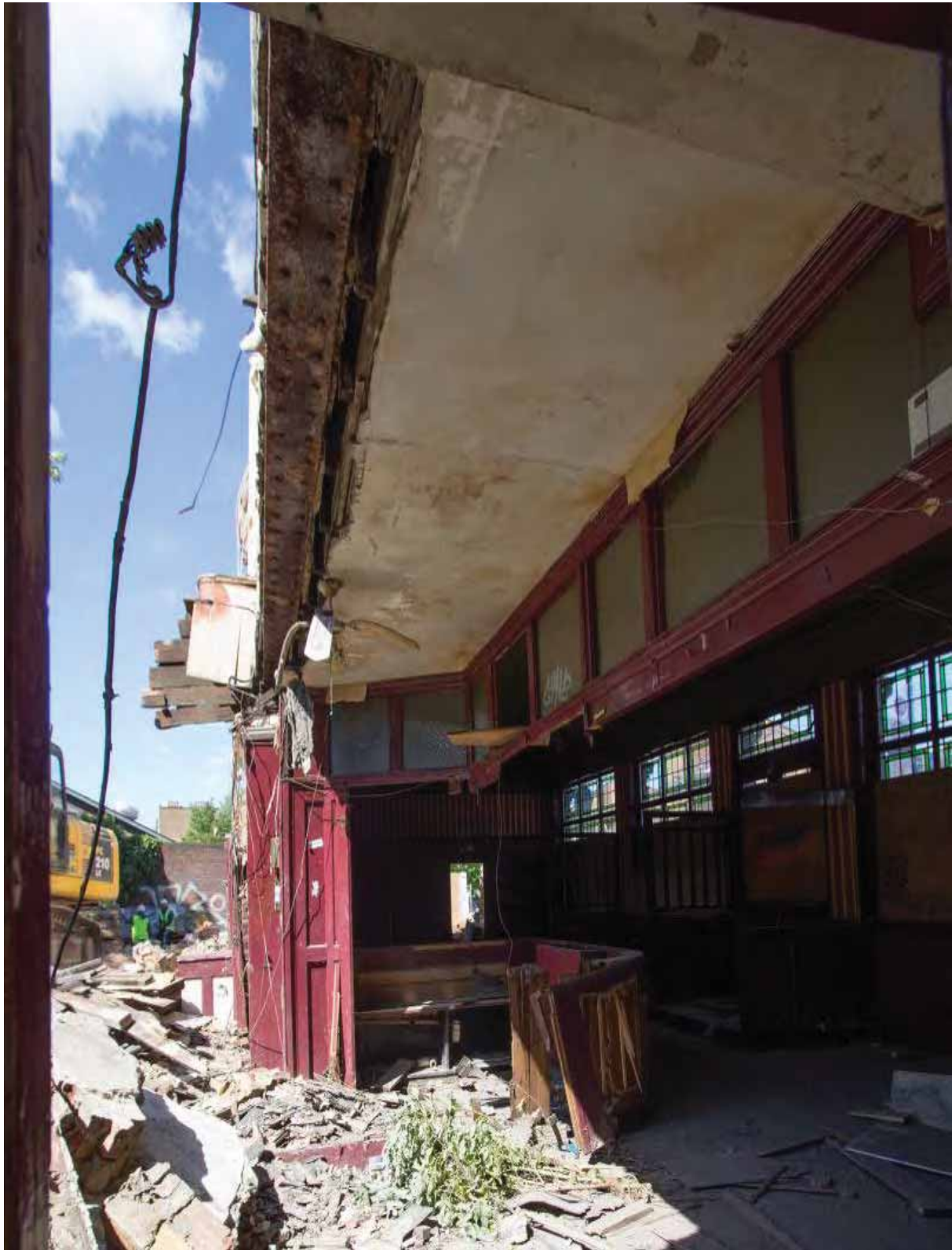
Plate 31 Composite iron beam at junction of eastern (Phase 2) and western (Phase 1) parts of the building, looking north
