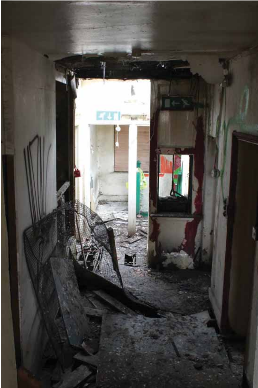
Plate 27 First floor corridor of the west (Phase 1) part of the building, showing dumb waiter, looking west
