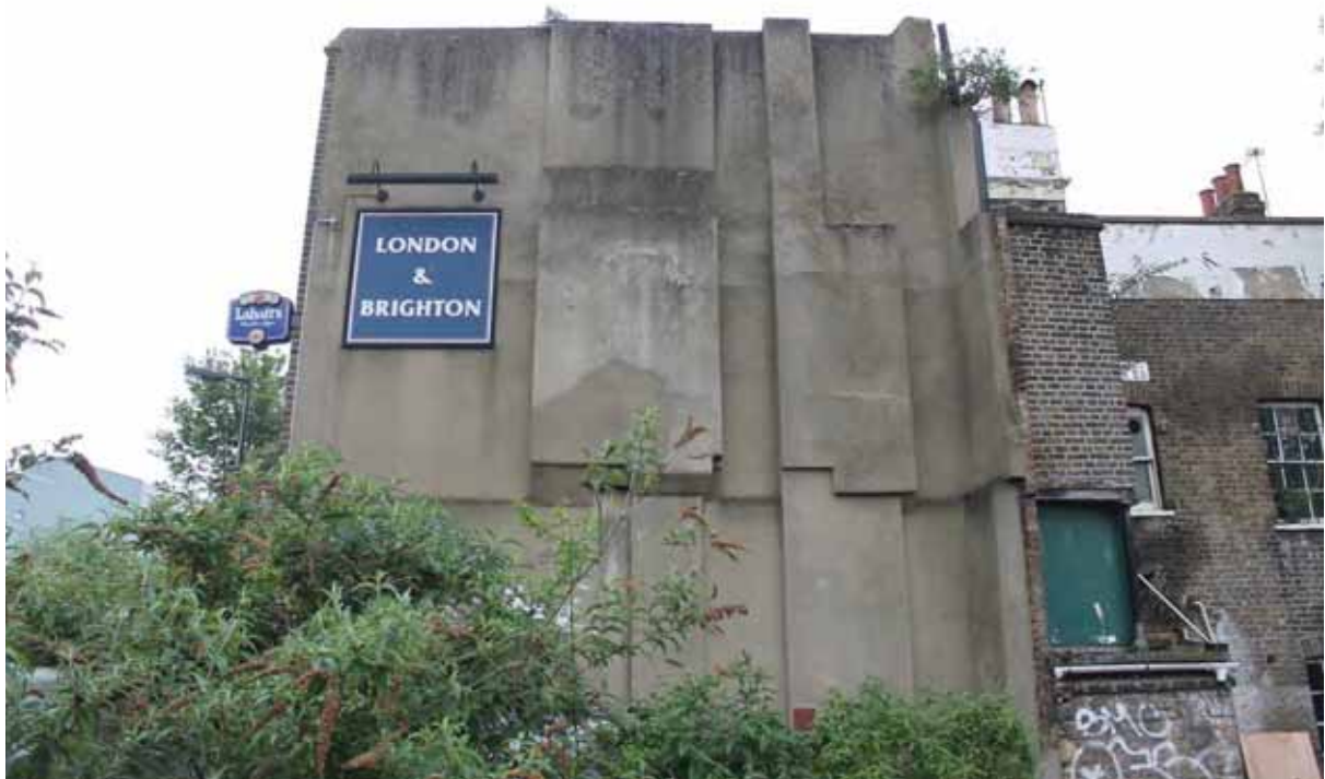
Plate 9 Rear northern rendered elevation of the eastern (Phase 2) part of the building, looking south
