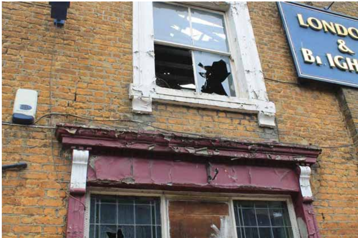
Plate 7 Inserted ground floor and original first floor window surrounds in the front (south) elevation of the west (Phase 1) part of the building, looking north
