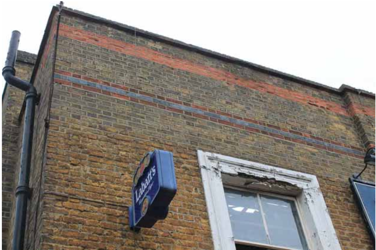
Plate 6 Southern elevation of the west Phase 1) part of the building showing earlier (lower) and later (upper) phases of brickwork, looking north
