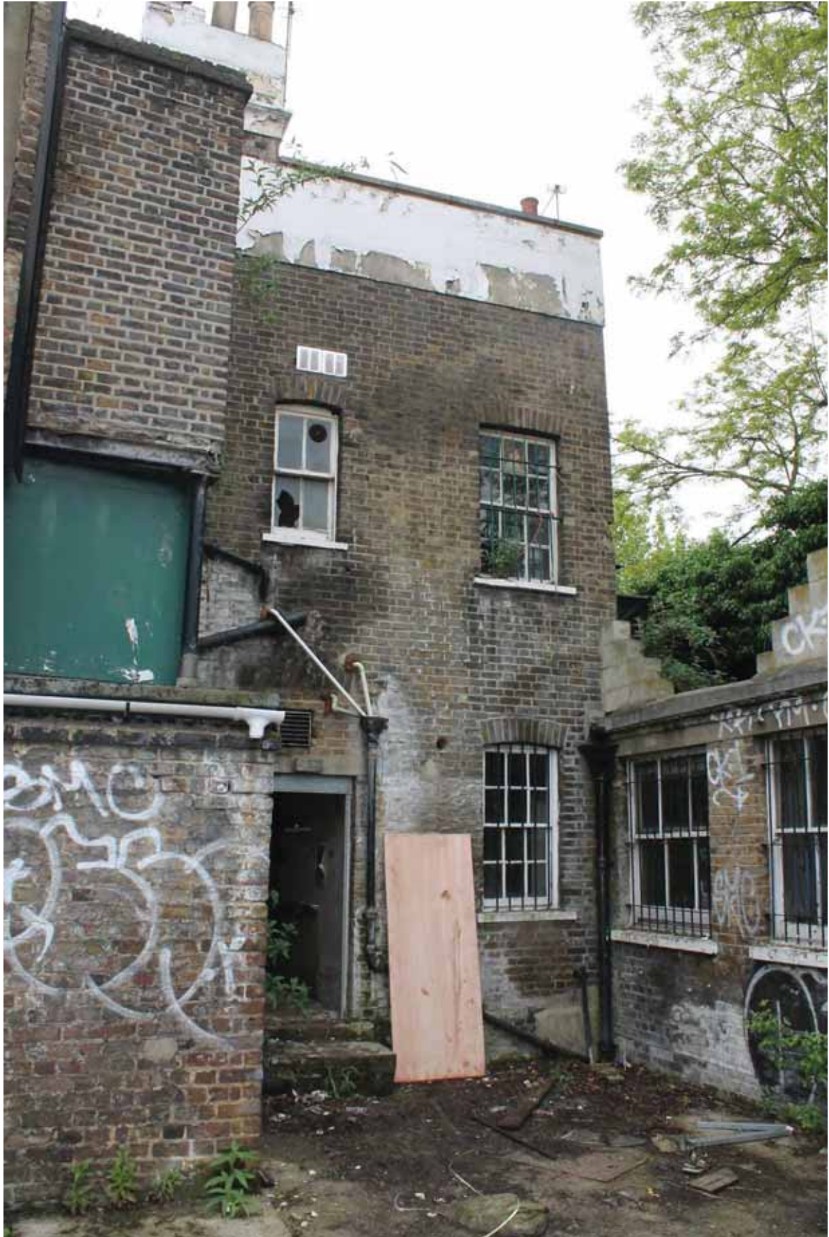
Plate 10 Rear (north) elevation of the western (Phase 1) part of the building (centre), looking south
