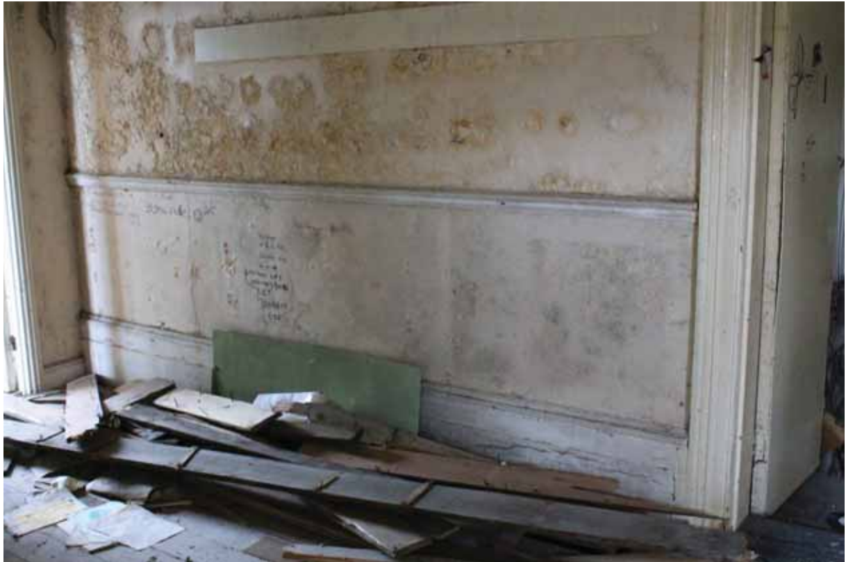
Plate 24 Original high skirting and dado along western wall of the first floor landing, looking west
