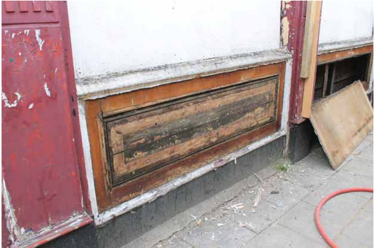
Plate 29 Circa 1890s oak panelling below ground floor window in the Asylum Road facade, looking north-west
