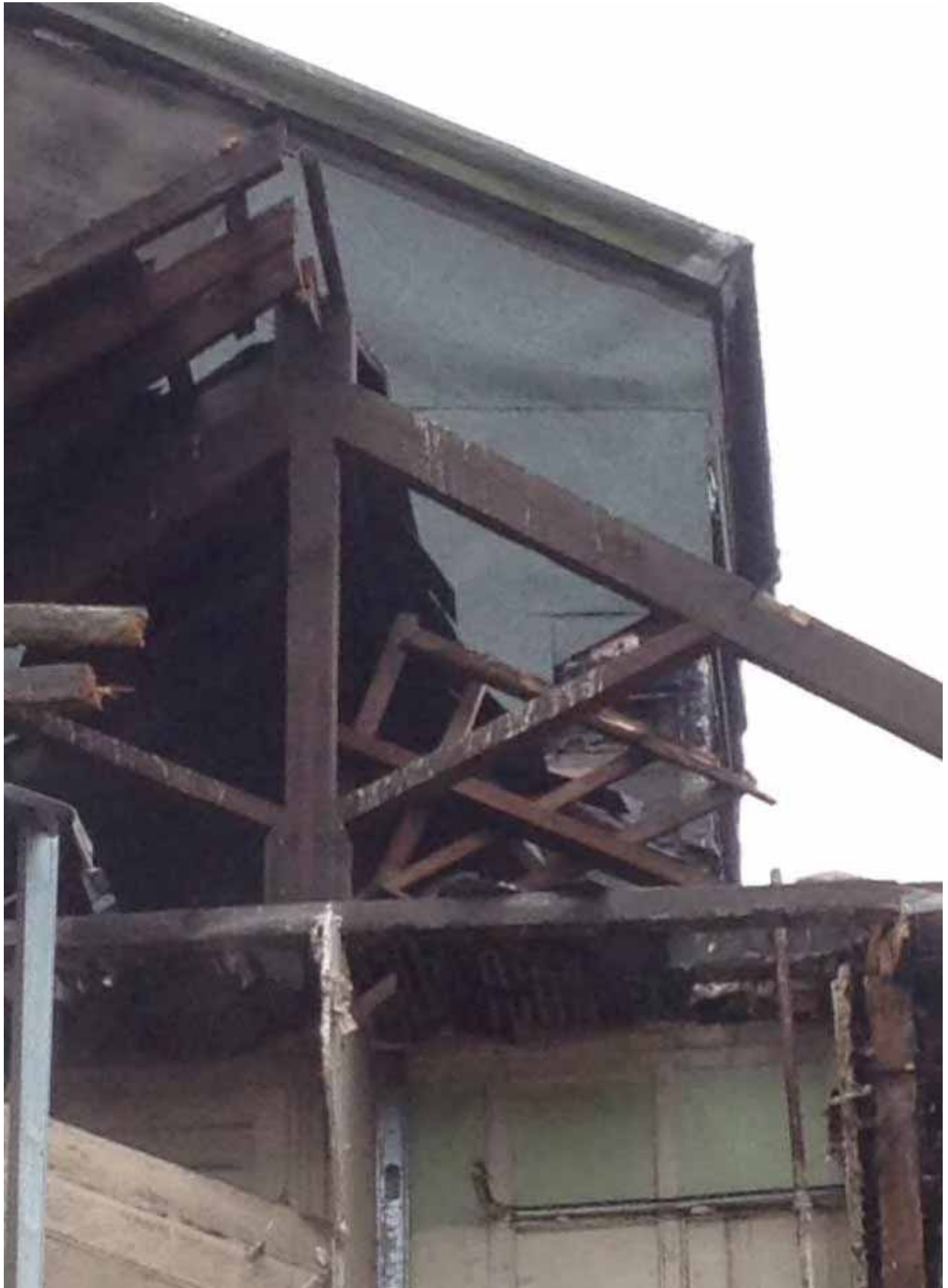
Plate 33 Staircase structure above the eastern pitched roof over the western (Phase 1) part of the building, looking south
