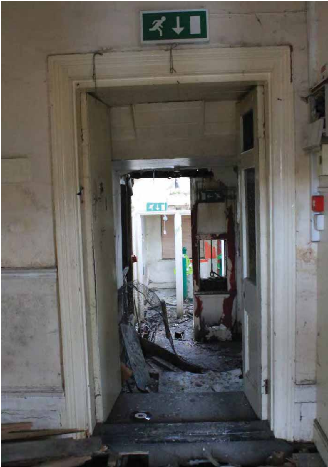
Plate 26 Doorway from the first floor landing into the west (Phase 1) part of the building, looking west
