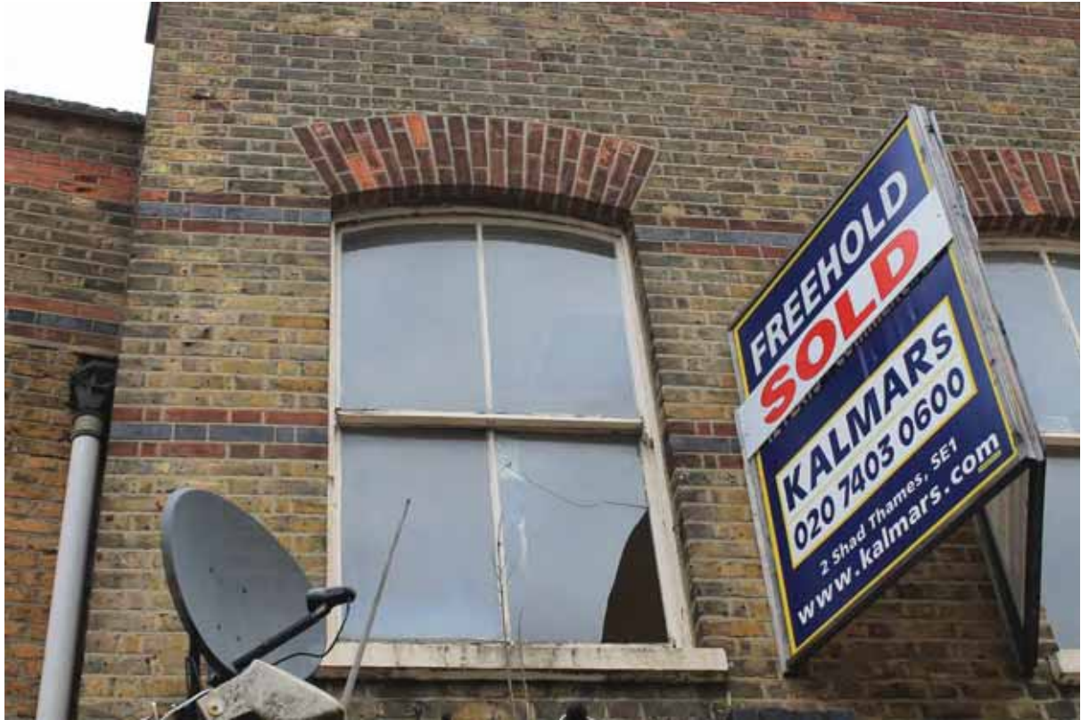
Plate 8 Detail of first floor window in the southern elevation of the eastern (Phase 2) part of the building
