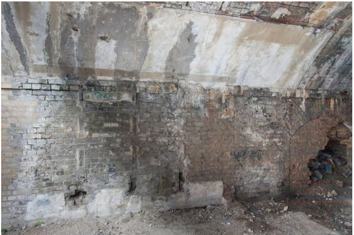
Plate 32 South end of the west wall in Arch 16 looking west (RWV13 D101 8335-2)
