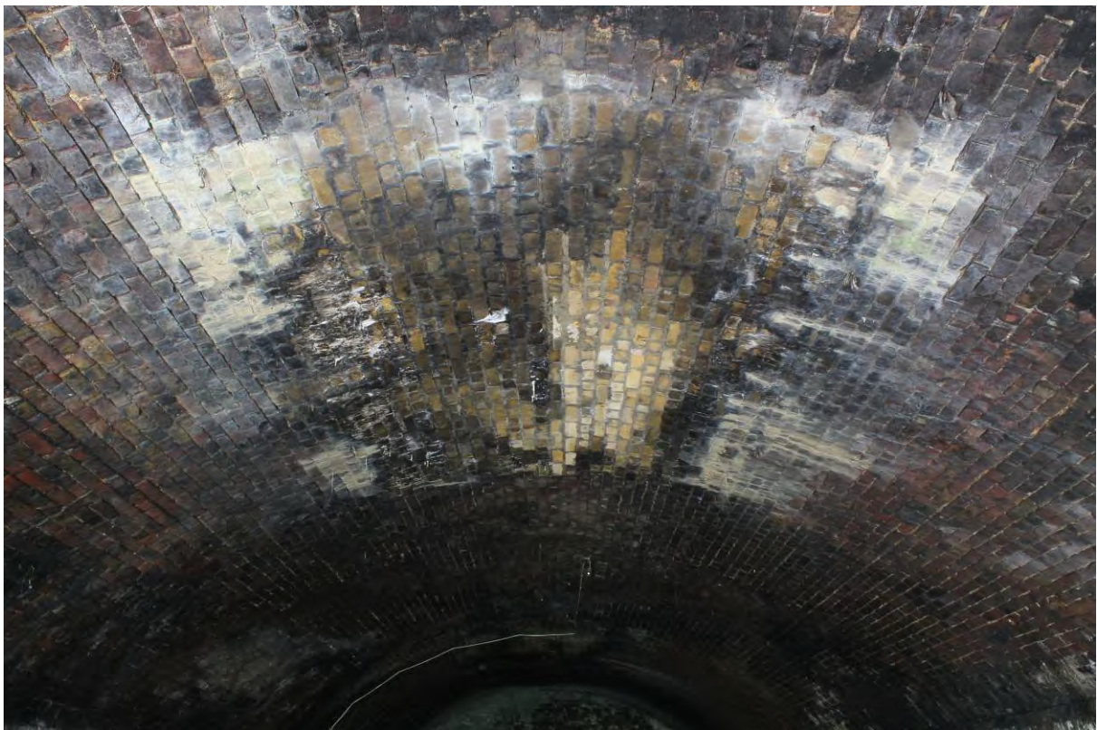
Plate 14 Arch 7 blocked coal drop
