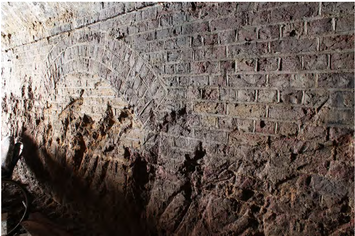
Plate 38 Damage to arch walls
