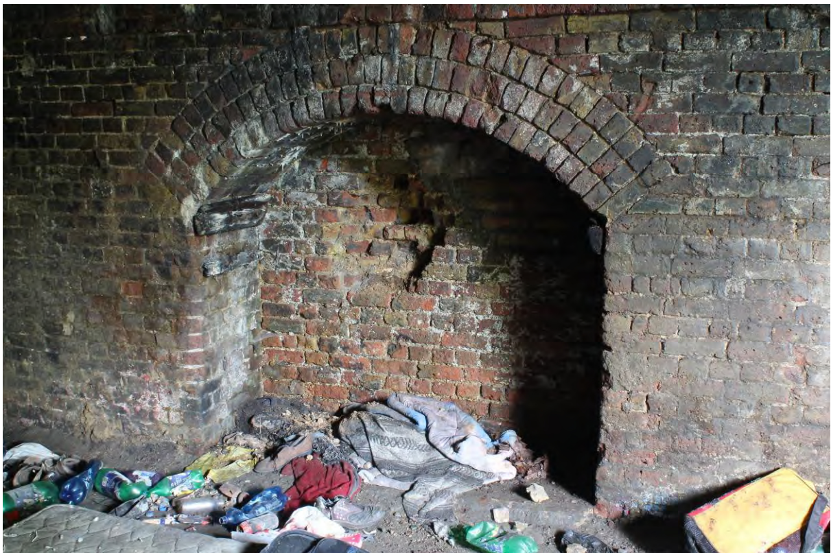
Plate 16 Blocked transverse arch within Viaduct Arch 8, looking north-east
