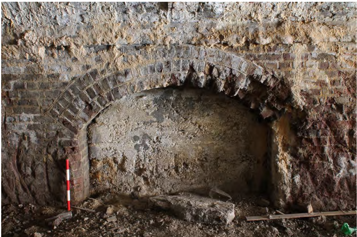
Plate 42 Damage to transverse arch in viaduct Arch 22
