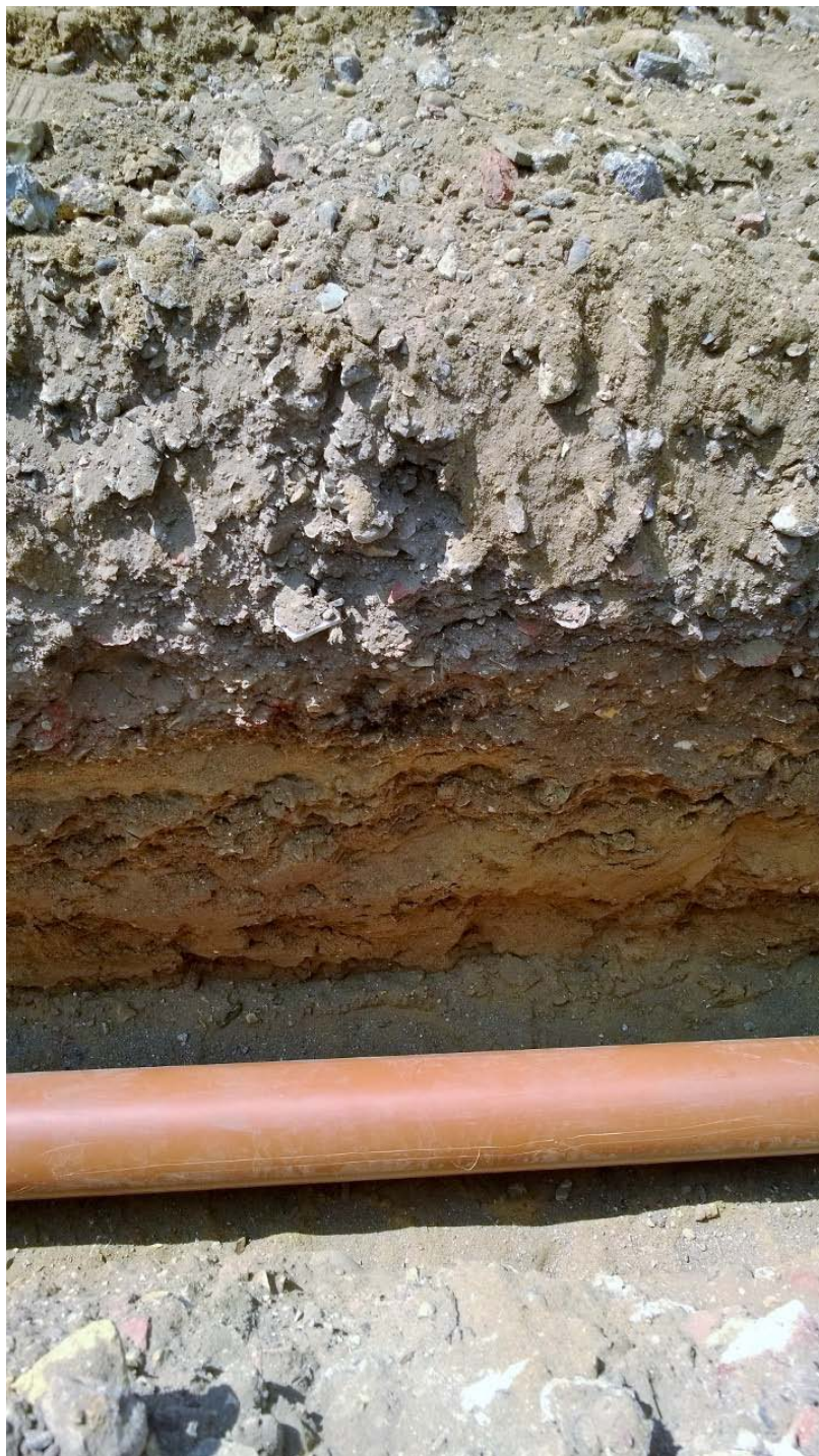
Plate 3: West facing view of section of service trench showing natural sands and gravels sealed by modern deposits
