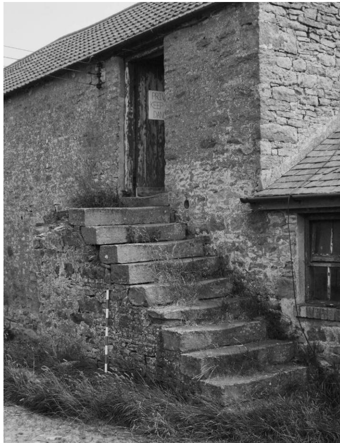
Photograph 15: Combination barn, west range, north part, steps to first floor on west side (scale 1m)
