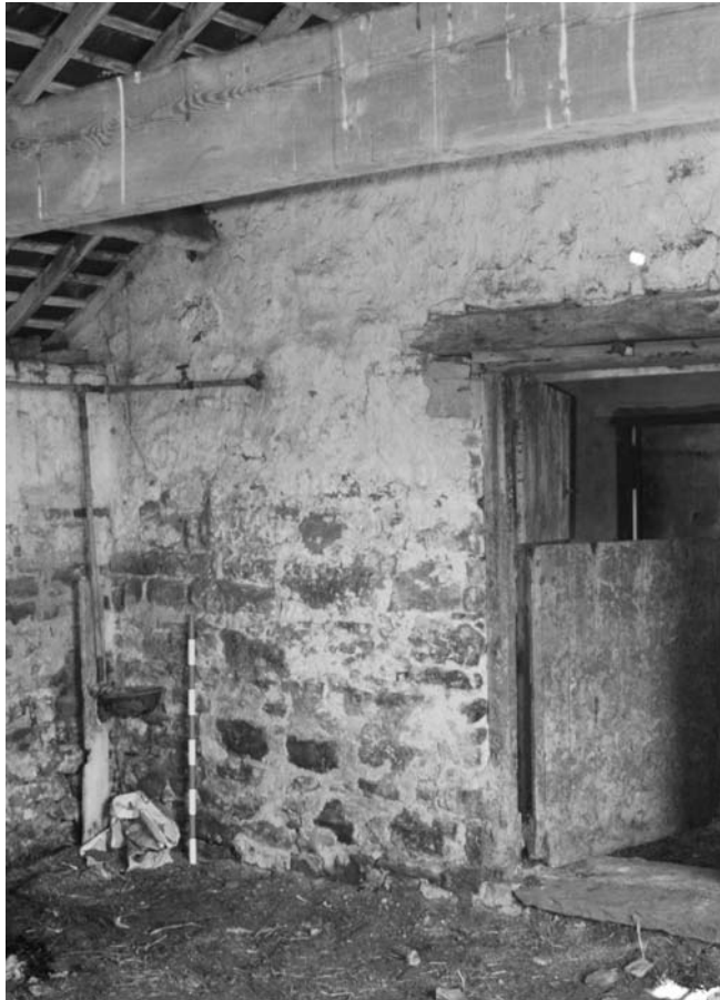
Photograph 25: Combination barn, west range, south part, north room interior, dividing wall (scale 1m)
