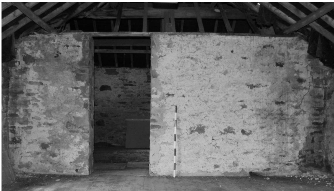
Photograph 18: Combination barn, north range, first floor, room interior, dividing wall (scale 1m)
