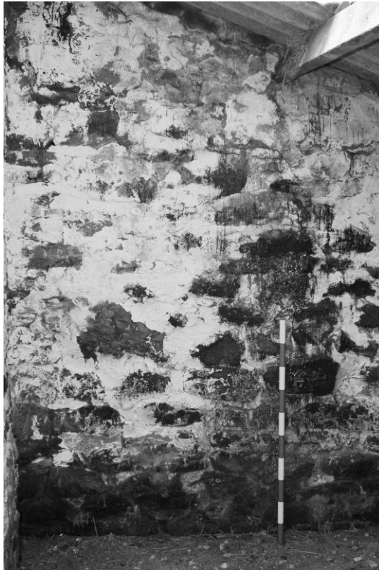
Photograph 36: Animal housing, north-west range, south-west room interior, end wall elevation (scale 1m)
