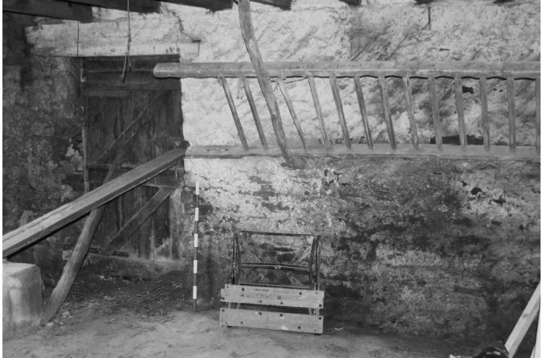
Photograph 21: Combination barn, west range, ground floor, north room interior, end wall (scale 1m)
