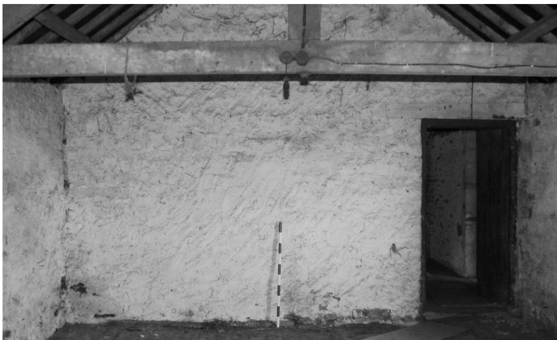
Photograph 16: Combination barn, west range, north part, first floor, south room interior, dividing wall (scale 1m)
