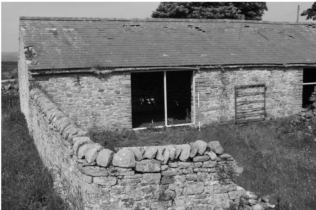
Photograph 10: Combination barn, west range, south part, east facing elevation (south portion) (oblique (scale 2m)
