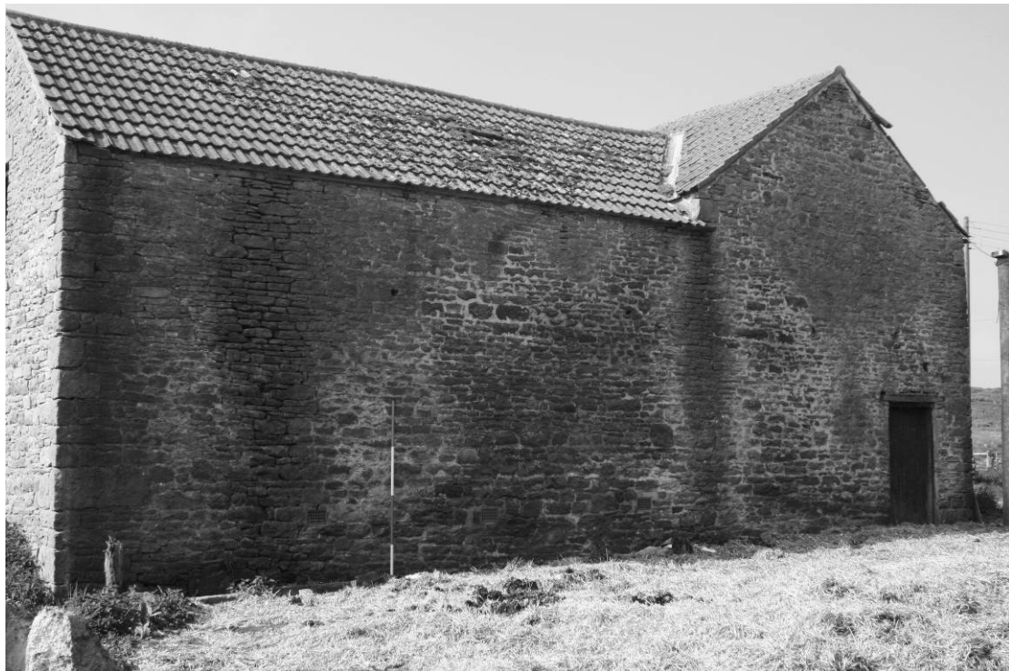
Photograph 2: Combination barn, north and west ranges, north facing elevation (oblique) (scale 2m)
