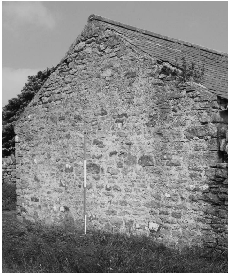
Photograph 12: Combination barn, west range, south part, south facing gable end elevation (oblique) (scale 2m)
