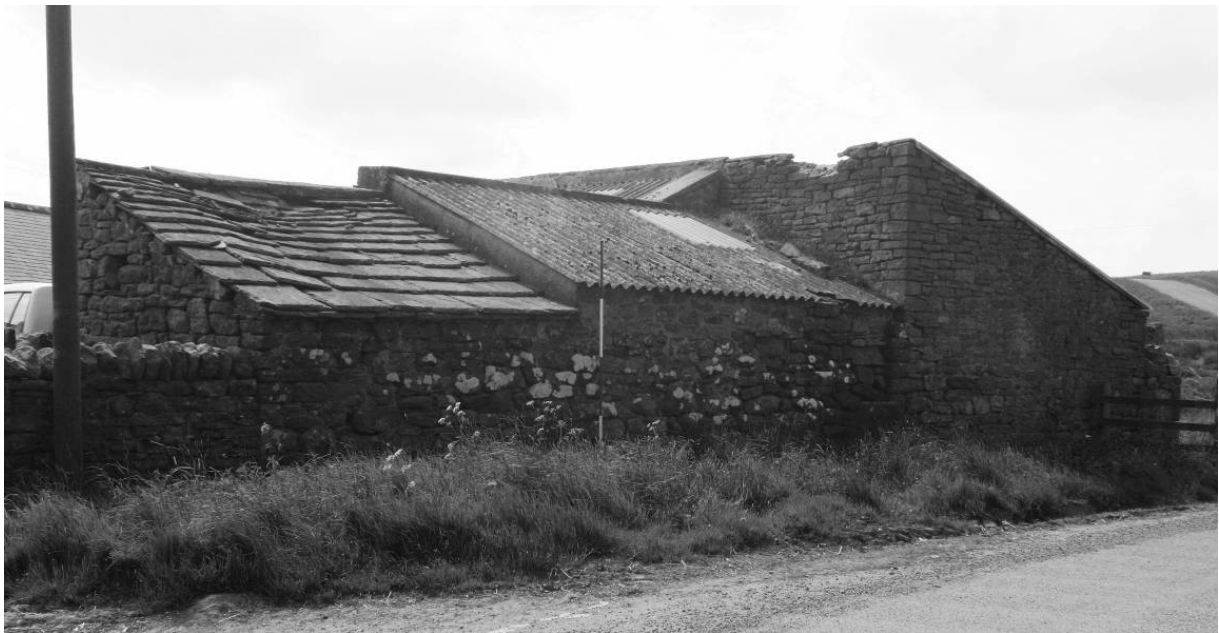
Photograph 34: Animal housing, north-west range, and lean-to barn, north-west facing elevation (oblique) (scale 2m)
