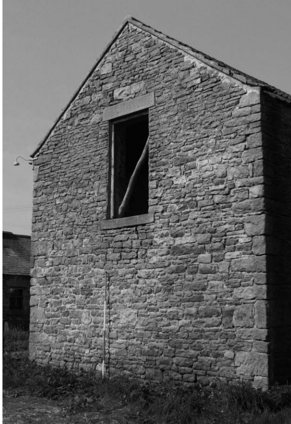
Photograph 3: Combination barn, north range, east facing gable end elevation (oblique) (scale 2m)
