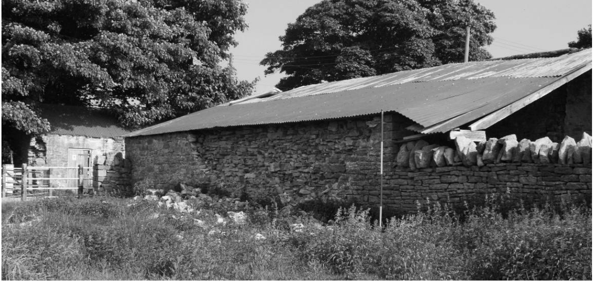
Photograph 31: Lean-to barn, south-west facing elevation (oblique), showing wall collapse (scale 2m)
