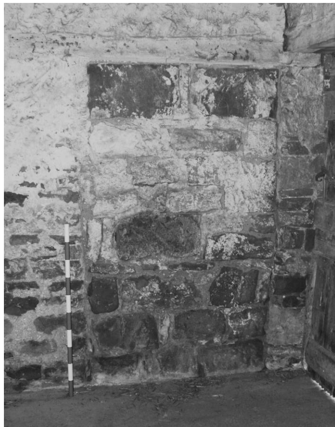
Photograph 22: Combination barn, west range, ground floor, north room interior, detail of infilled doorway (scale 1m)
