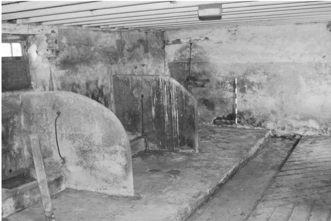
Photograph 23: Combination barn, west range, north part, ground floor, stable room interior (scale 1m)
