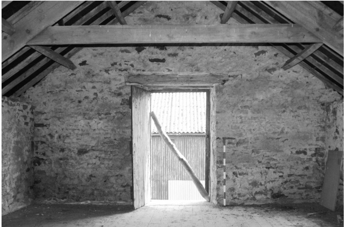
Photograph 19: Combination barn, north range, first floor, room interior, gable end wall (scale 1m)
