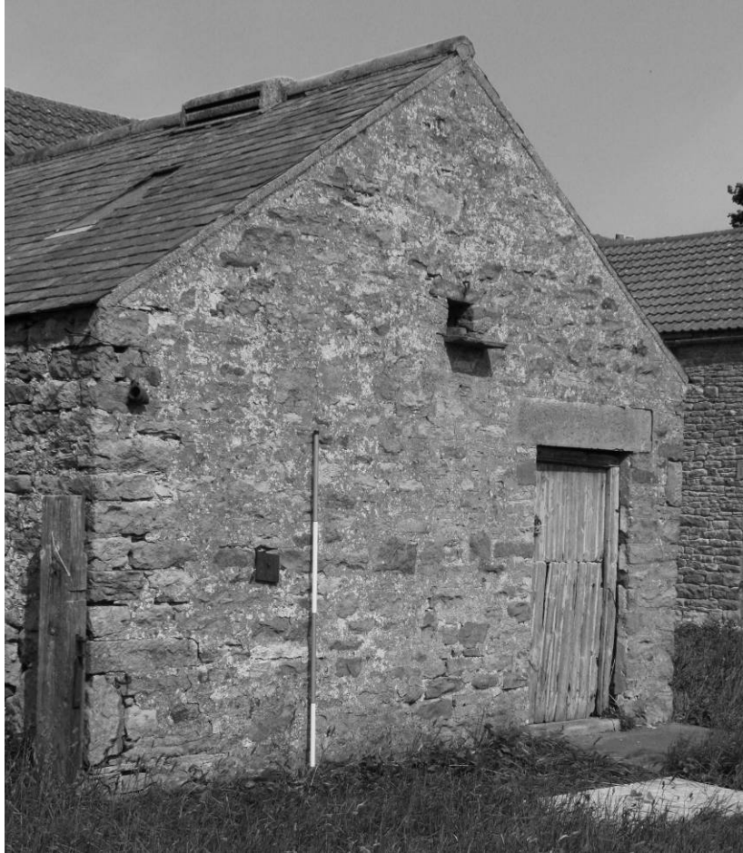
Photograph 7: Combination barn, south range, east facing gable end elevation (oblique) (scale 2m)
