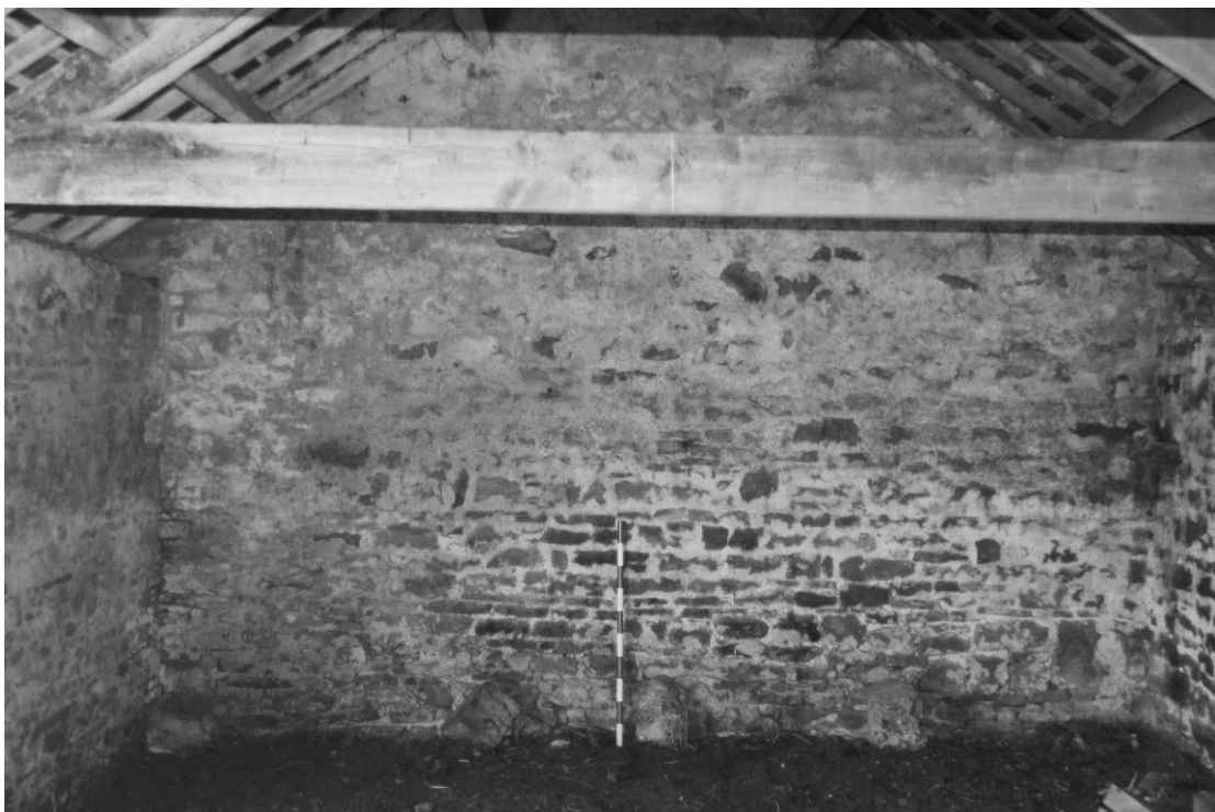
Photograph 26: Combination barn, west range, south part, south room interior, end wall (scale 1m)
