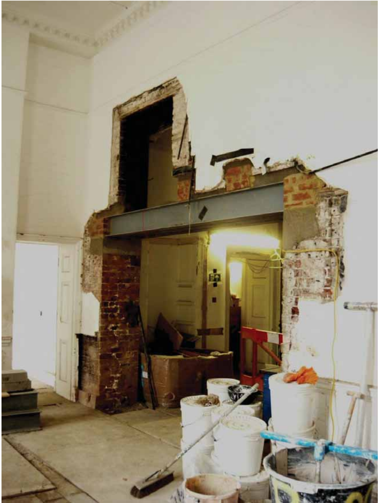
Plate 349: North (left) and east (right) walls in Room G01, looking north-east (EAF10 BHD8 (122))
