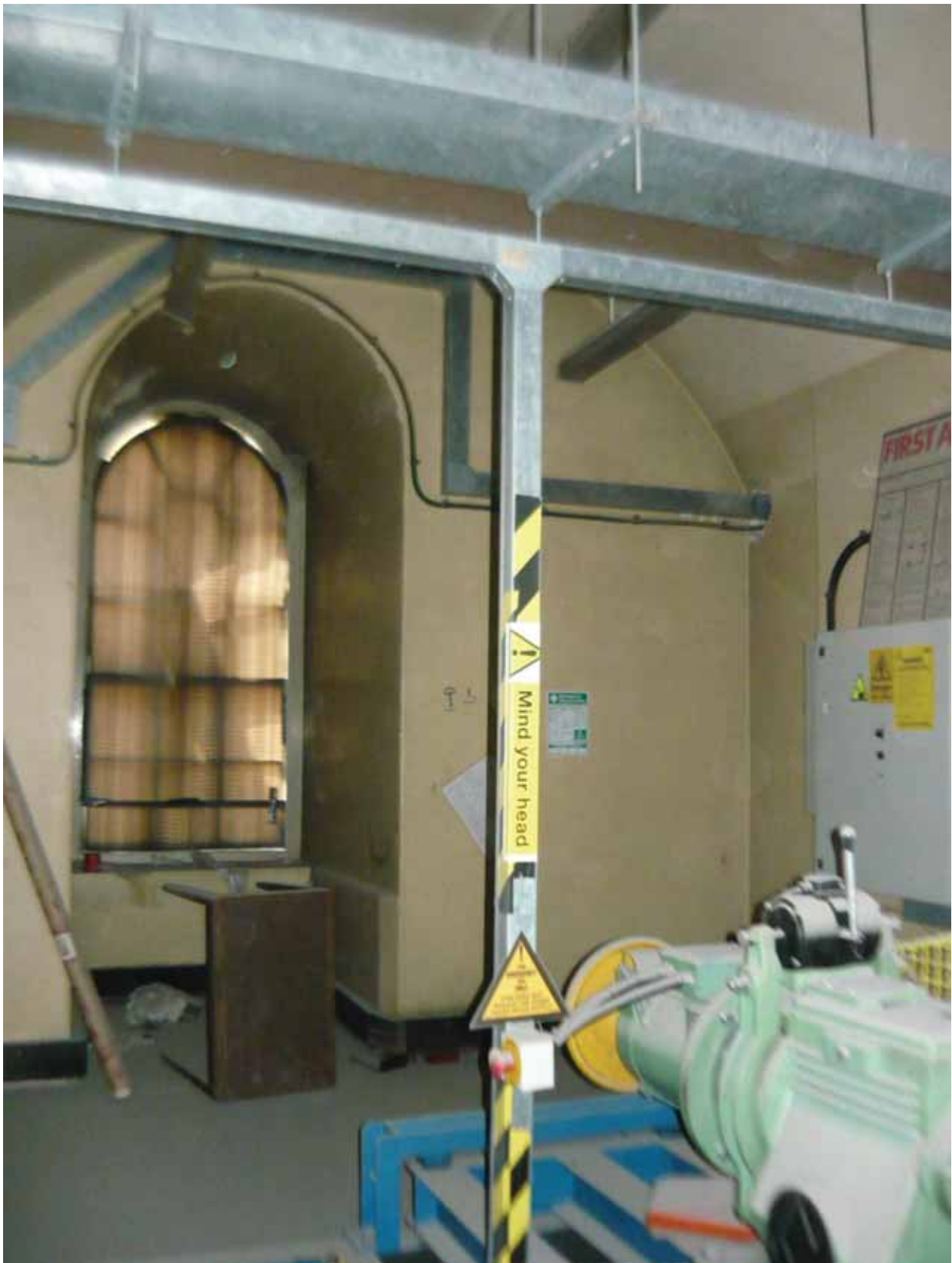
Plate 193: Window in the west wall of Room M114, looking west (EAF10 BHD2 (111))
