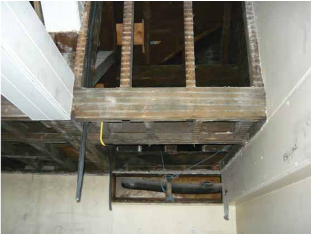
Plate 678: Exposed roof structure and lead pipe at the south end of Room T03, looking east (EAF10 BHD10 (62))
