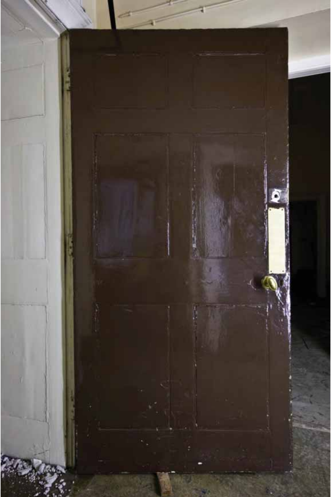
Plate 261: Doorway in the east wall of Cupboard 02LG looking south (EAF10 LG100 0989)
