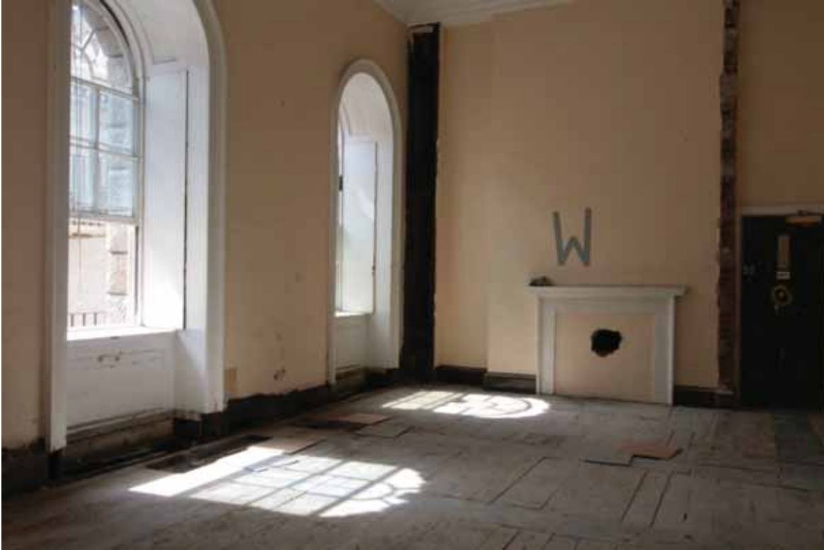
Plate 203: West (left) and north (right) walls of Room M16, looking north-west (EAF10 311)
