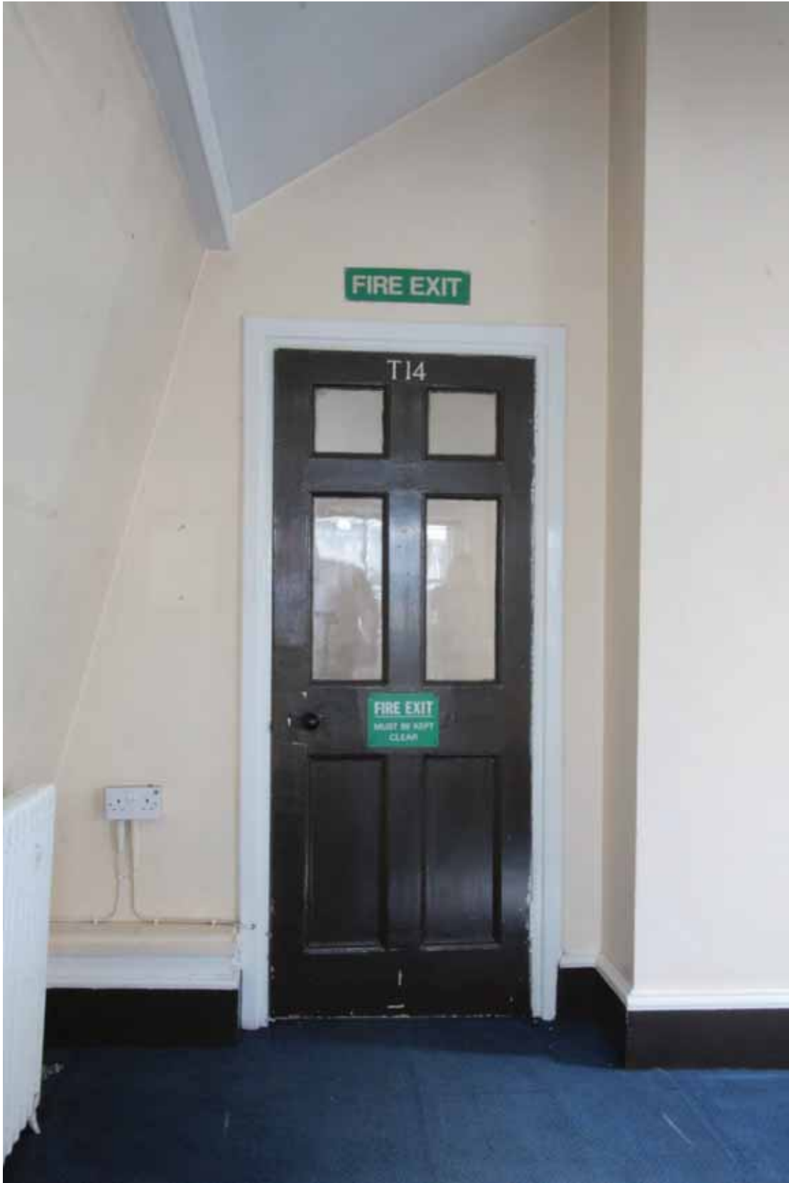
Plate 694: Doorway at the north end of the east wall in Room T09, looking east (EAF10 1)
