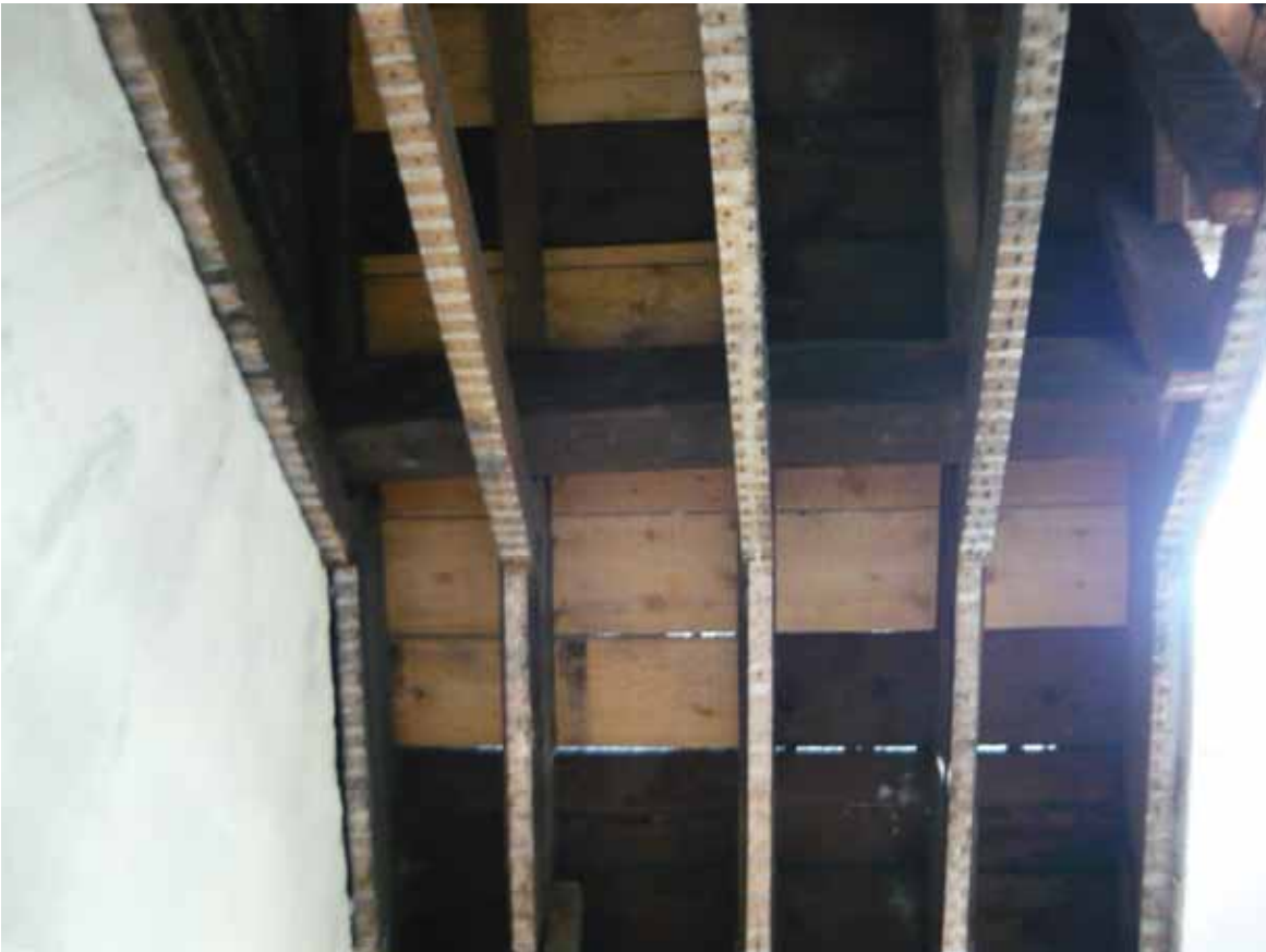
Plate 752: South end of the west side of the roof over Room T17, looking west (EAF10 BHD10 (23))
