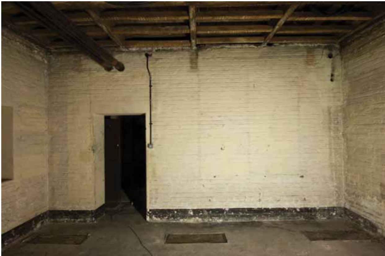
Plate 131: North wall of Room B52, looking north (DSC_1439 _sitecode EAF10_© PCA Ltd 2010)
