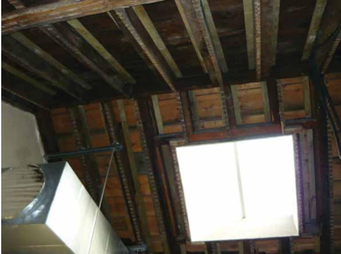
Plate 692: Skylight at the north end of the east side of the roof above Room T08, looking east (EAF10 BHD10 (75))
