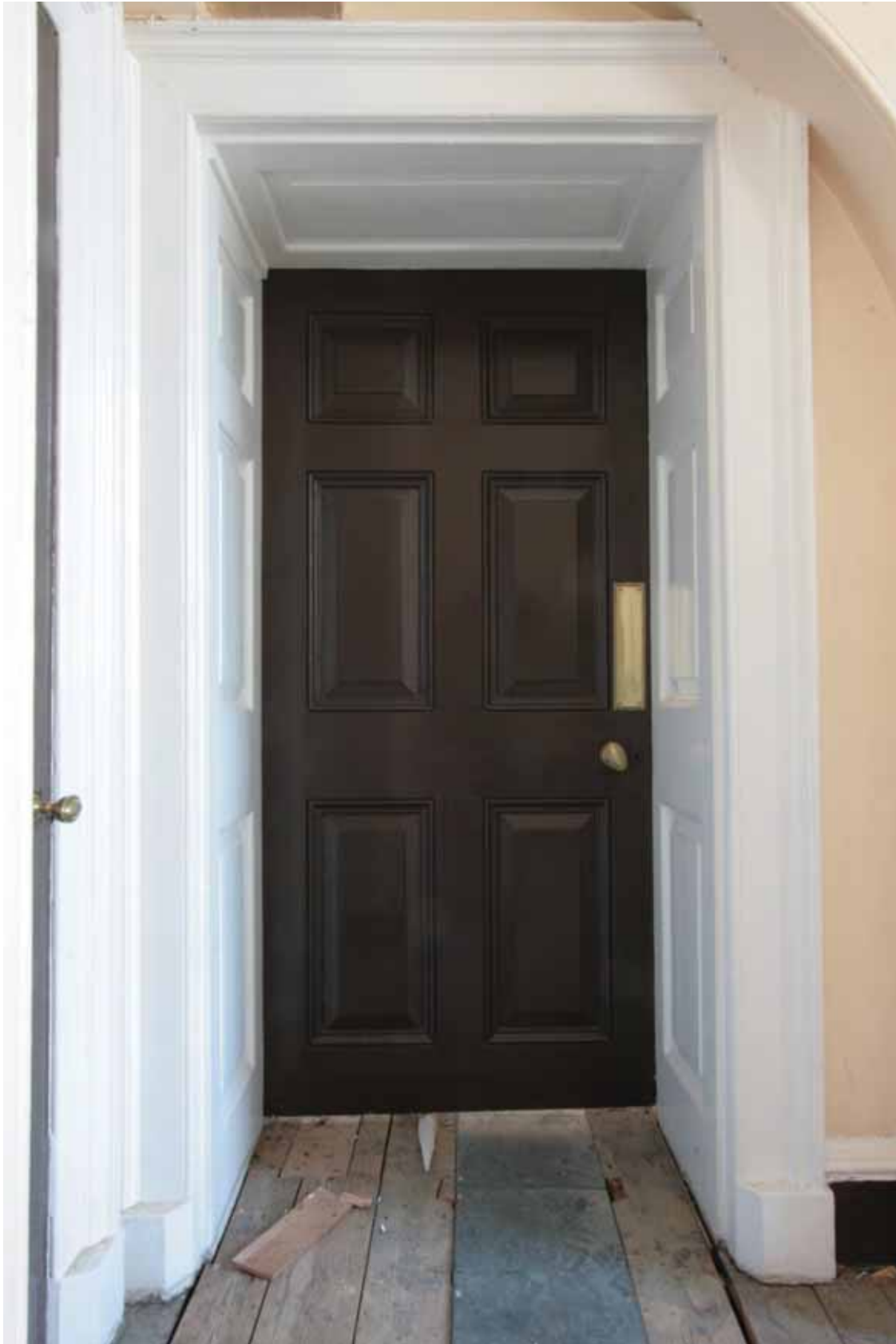
Plate 457a: Doorway in the south wall of Room F67, looking south (EAF10 170)
