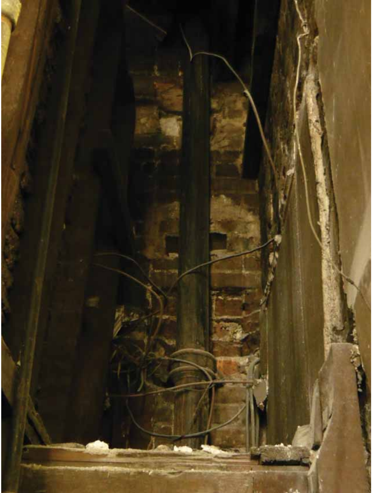
Plate 522: Void at the north end of the partition wall in Room F16, looking up and west (EAF10 BHD8 (33))
