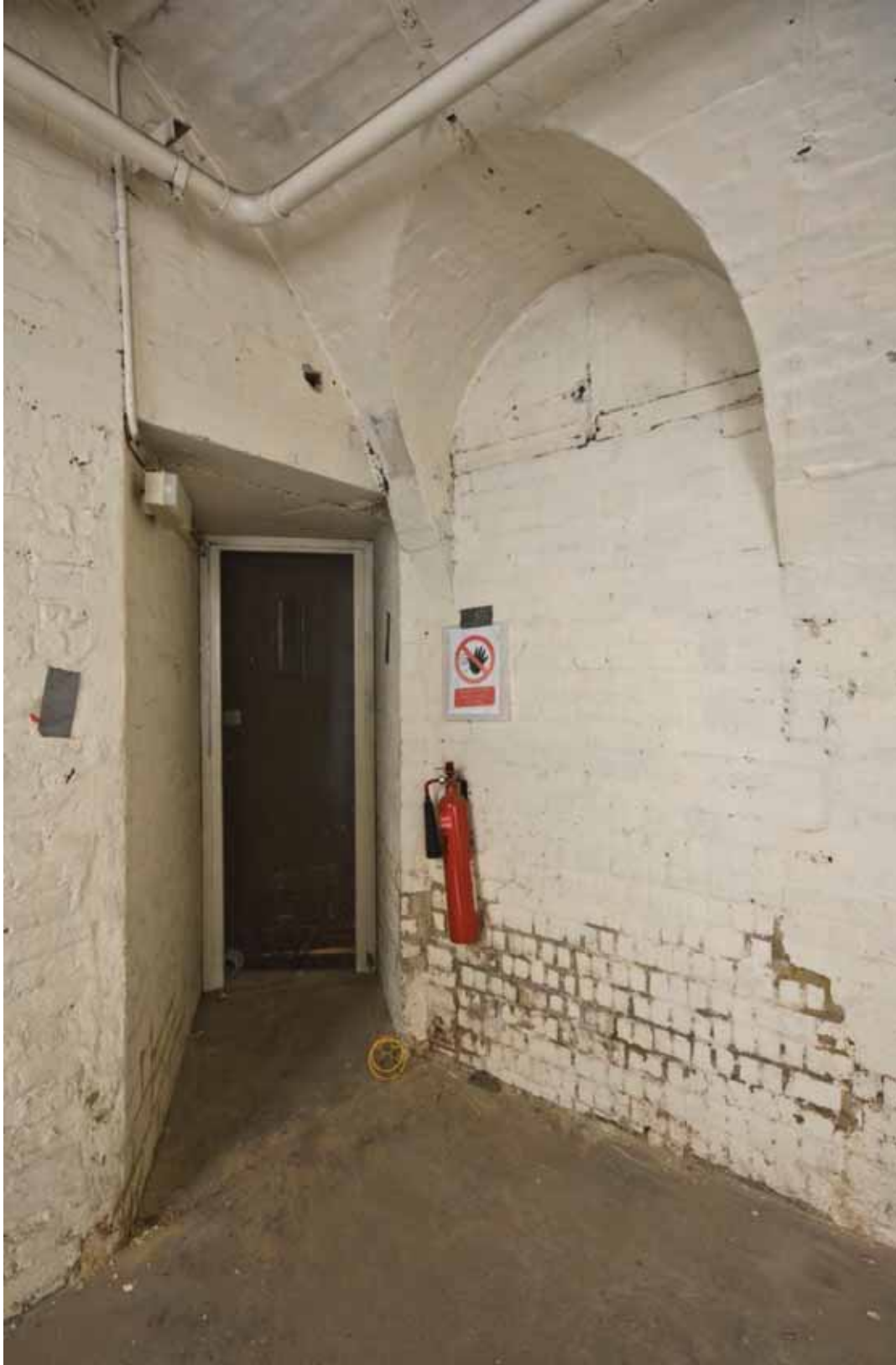
Plate 125: Doorway at the west end of the south wall and blocked doorway (right) at the south end of the west wall in Room B50, looking south-west (DSC_1362 _sitecode EAF10_© PCA Ltd 2010 _2)
