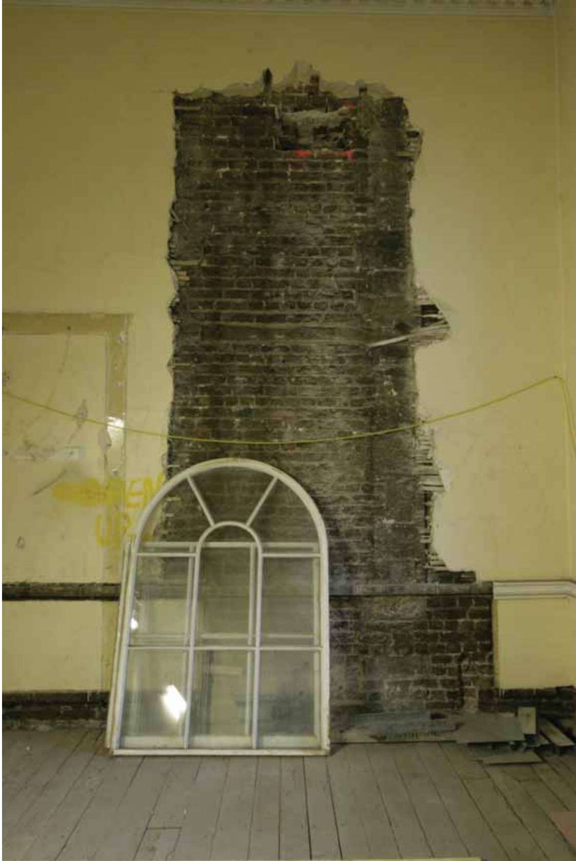
Plate 451: Area of removed plaster from the north wall of Room G28, looking north (EAF10 A100 026)
