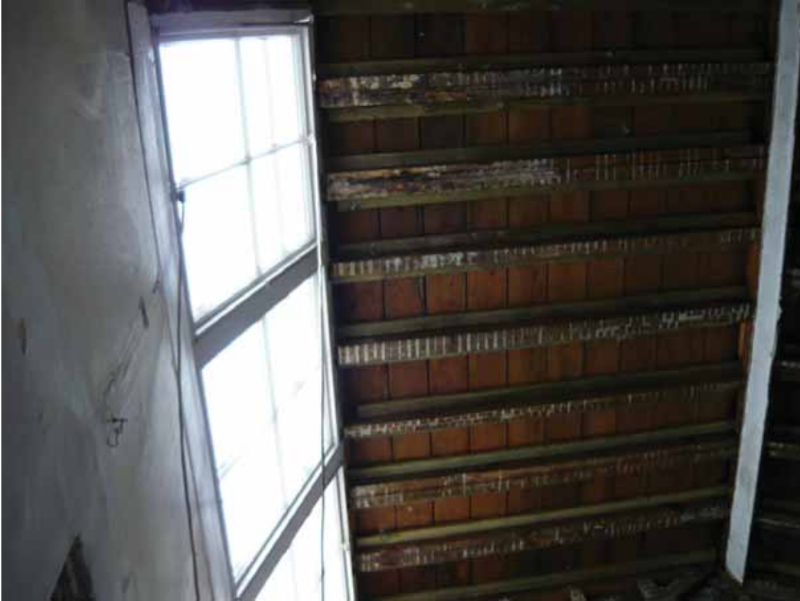
Plate 775: Dormer window in the west side of the roof above Room T24 (EAF10 BHD10 (13))
