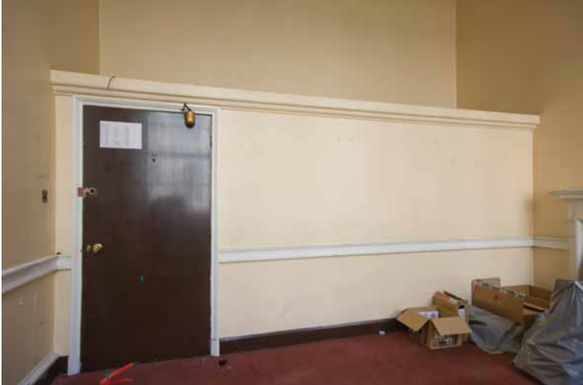
Plate 445: South (left), west partition (centre) and north (right) walls in Room G27, looking west (EAF10 B100 0936)
