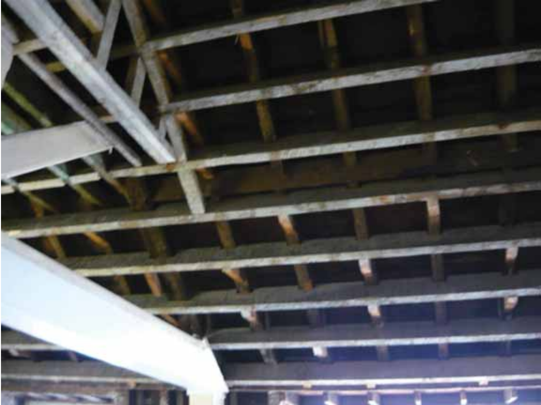
Plate 738: Roof structure above the east wall of Room T117, looking east (EAF10 BHD10 (39))
