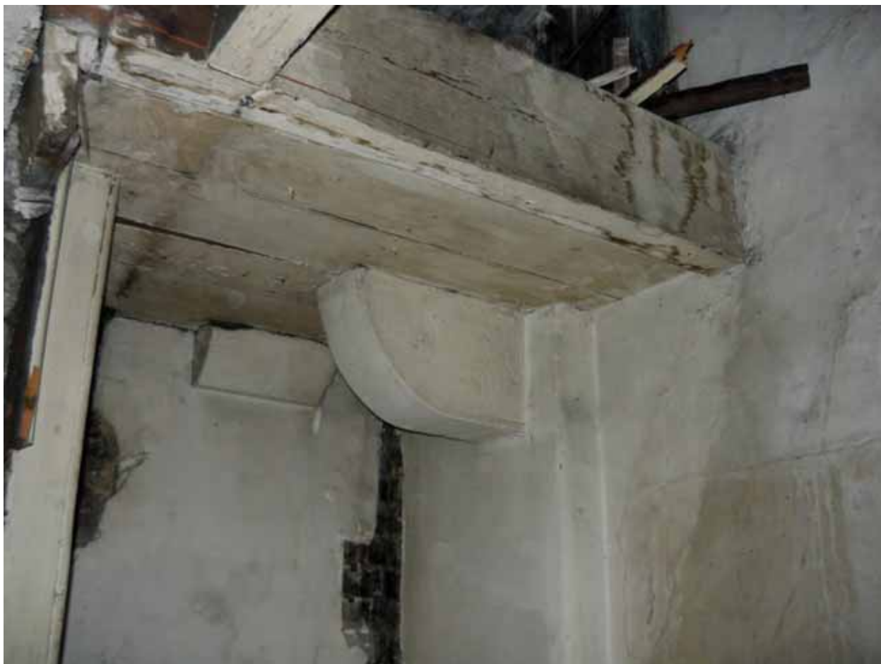
Plate 222: Stone corbels supporting landing/mezzanine in south-west corner of Room M18, looking south-west (EAF10 BHD6 (31))
