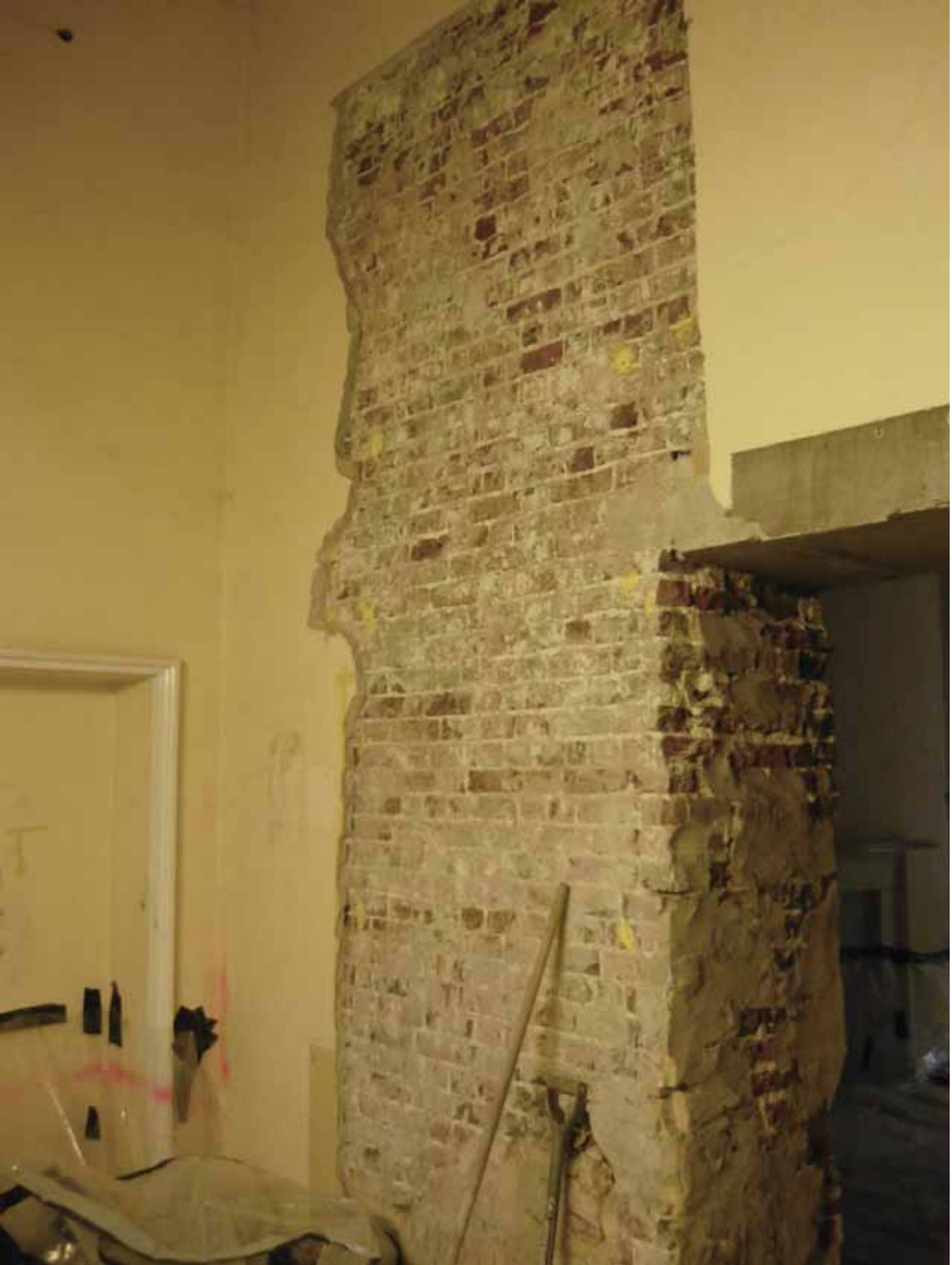
Plate 239b: Stripping of plaster from the south side of the west doorway in Corridor 05LG looking west (EAF10 BHD6 (21))
