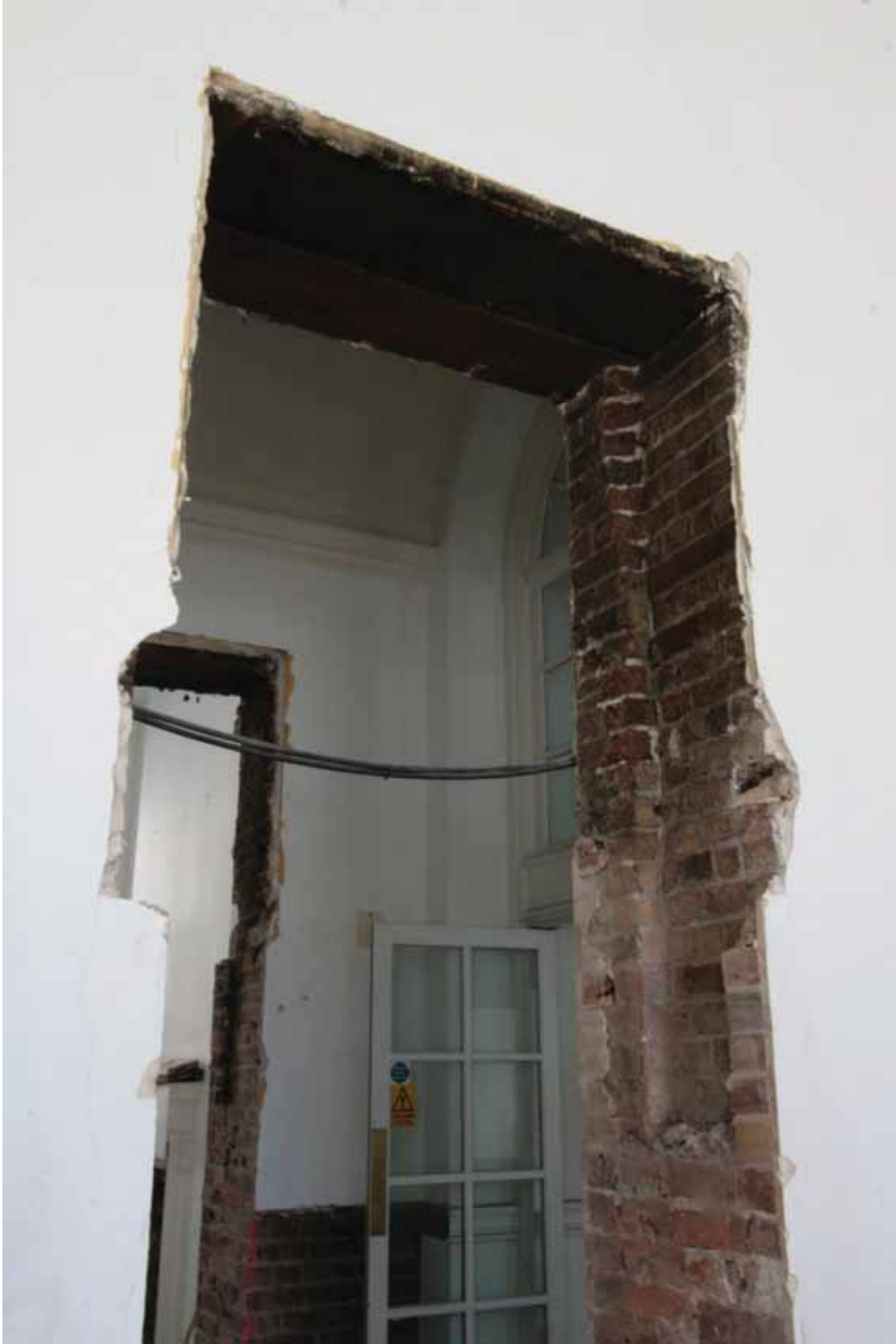
Plate 368: New doorway cut through the south end of the east wall in Room G08 in 2010, looking south-east (EAF10 268)
