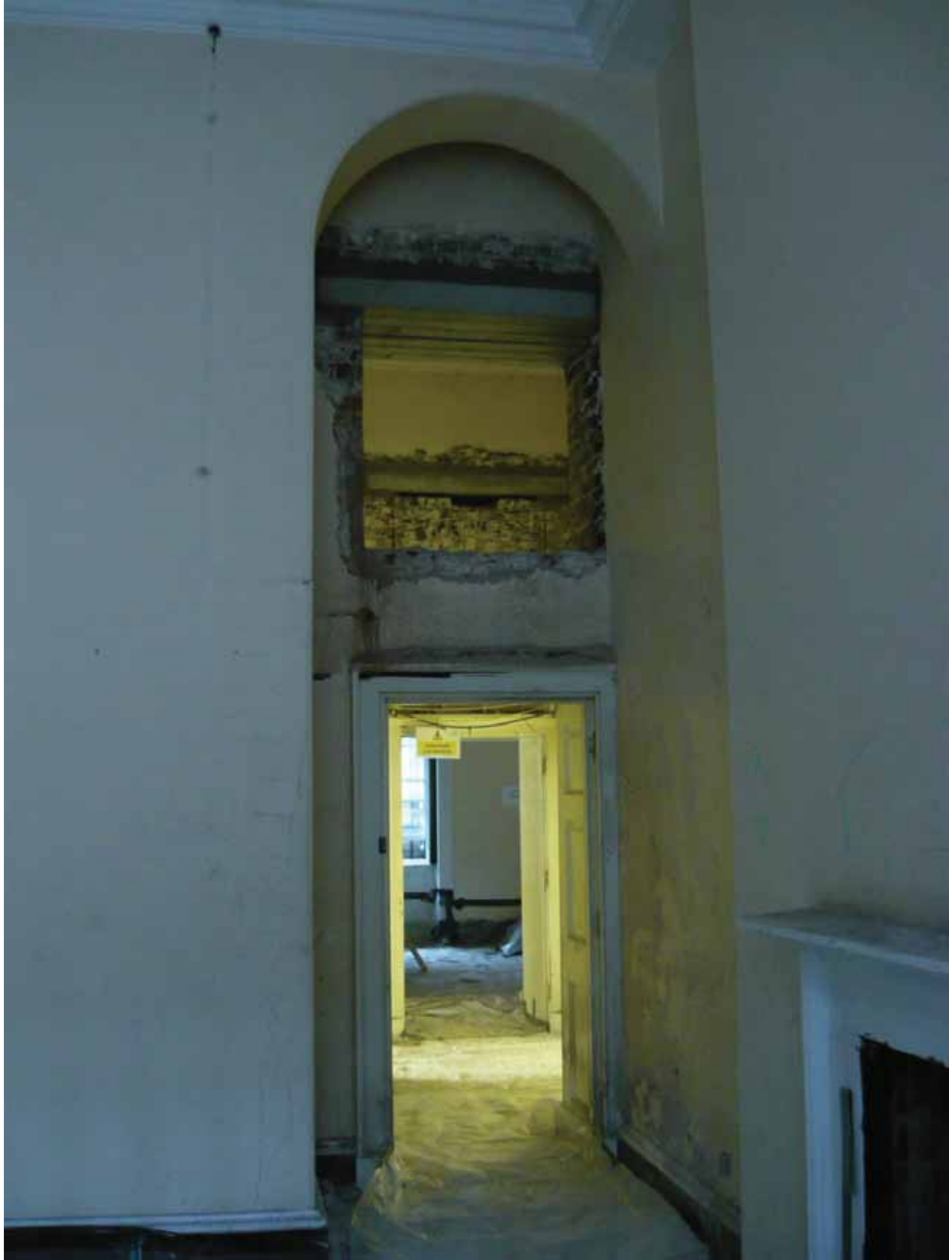
Plate 181: East (left) and south (right) walls of Room M09, looking east (EAF10 BHD6 (104))
