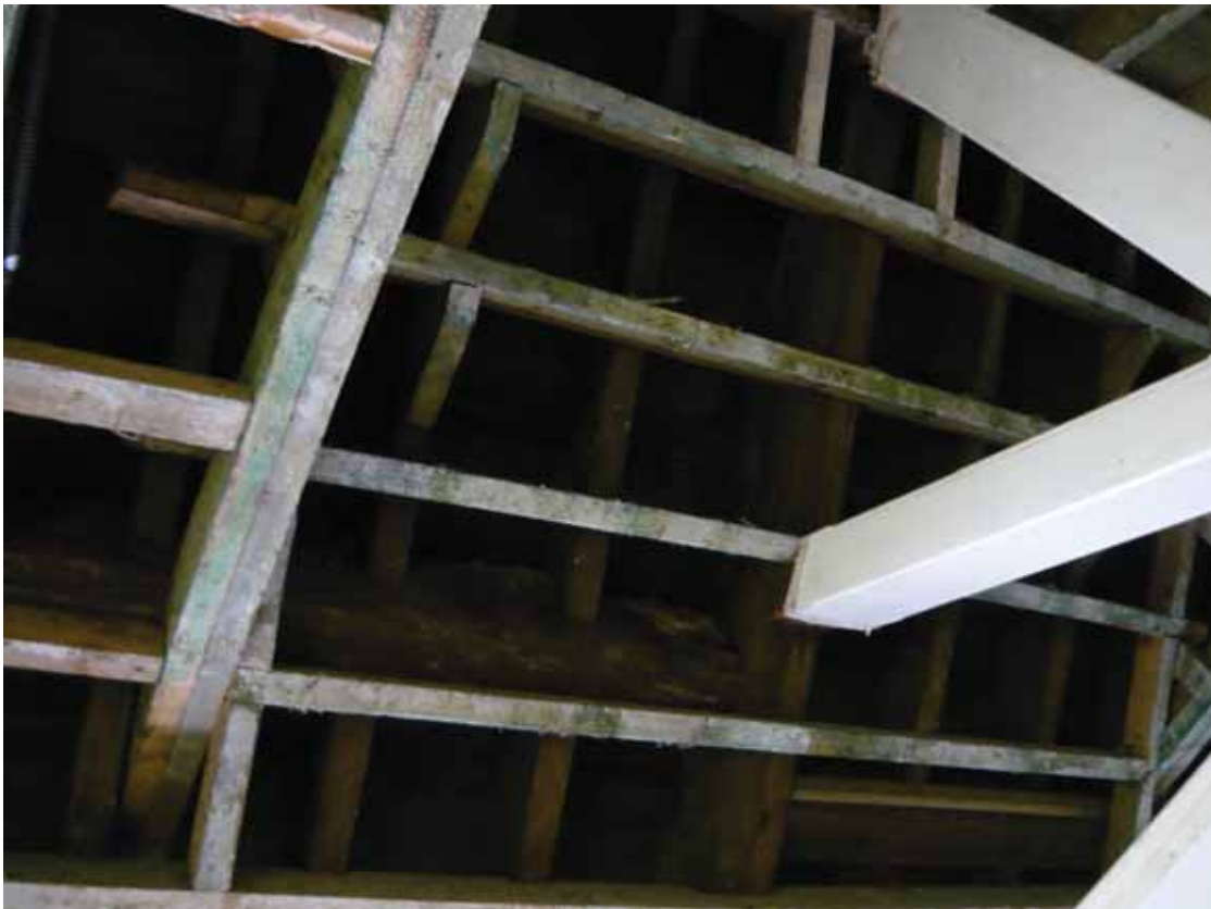
Plate 731: Roof structure above the east wall in Room T115, looking south-east (EAF10 BHD10 (43))
