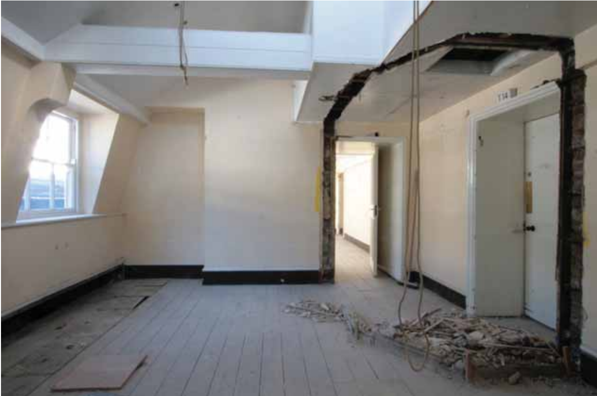
Plate 787: East (left), south (centre) and west (right) walls in Room T28, looking south (EAF10 213)
