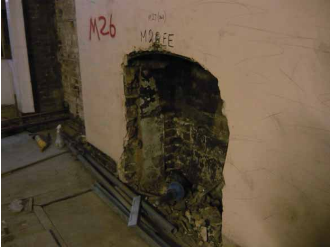
Plate 307: Fireplace in the south wall in Room M26/M27, looking south-east (EAF10 BHD13 (4))
