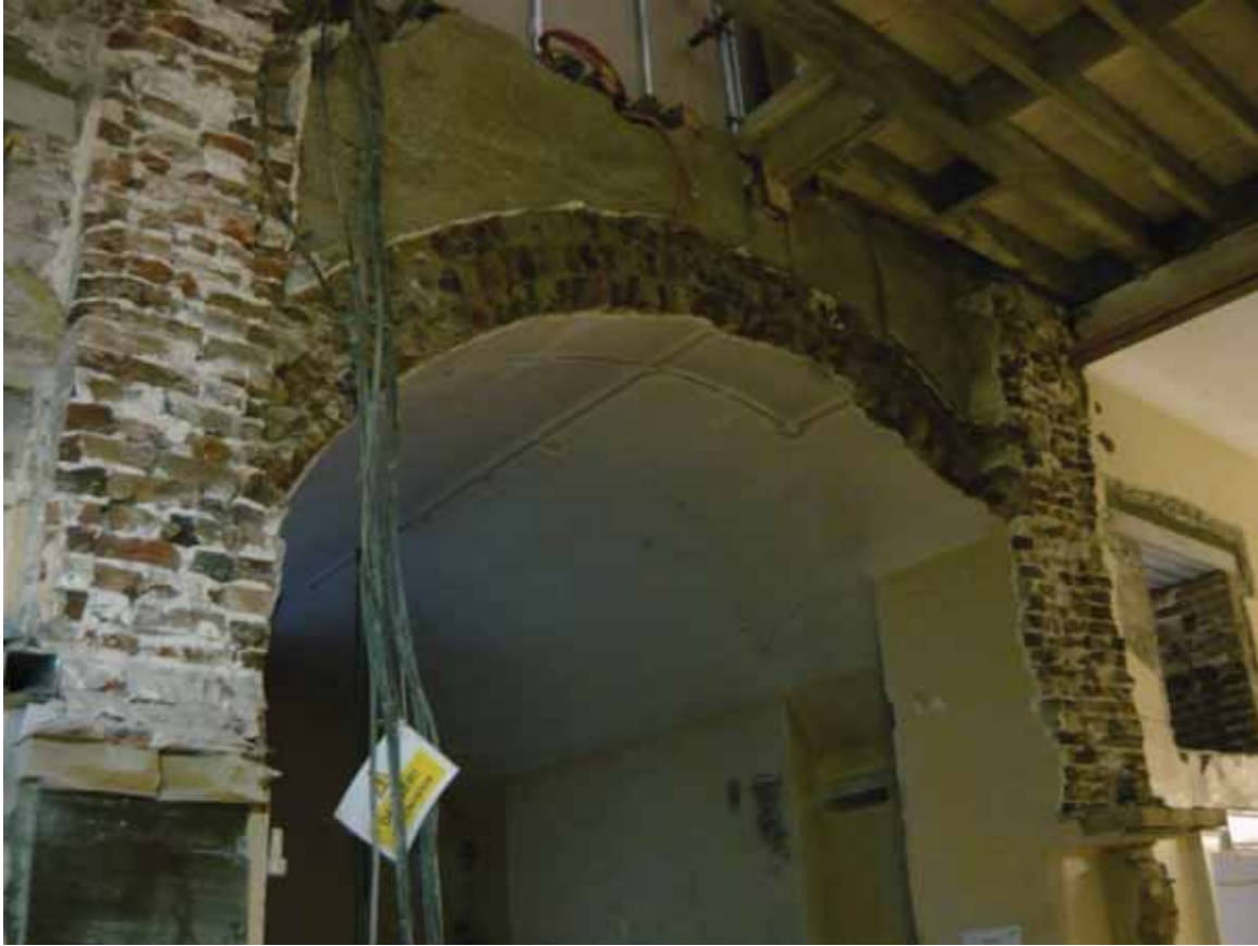
Plate 194b: Brick barrel vaulted ceiling in Room M114, looking north-west (EAF10 BHD13 (5))
