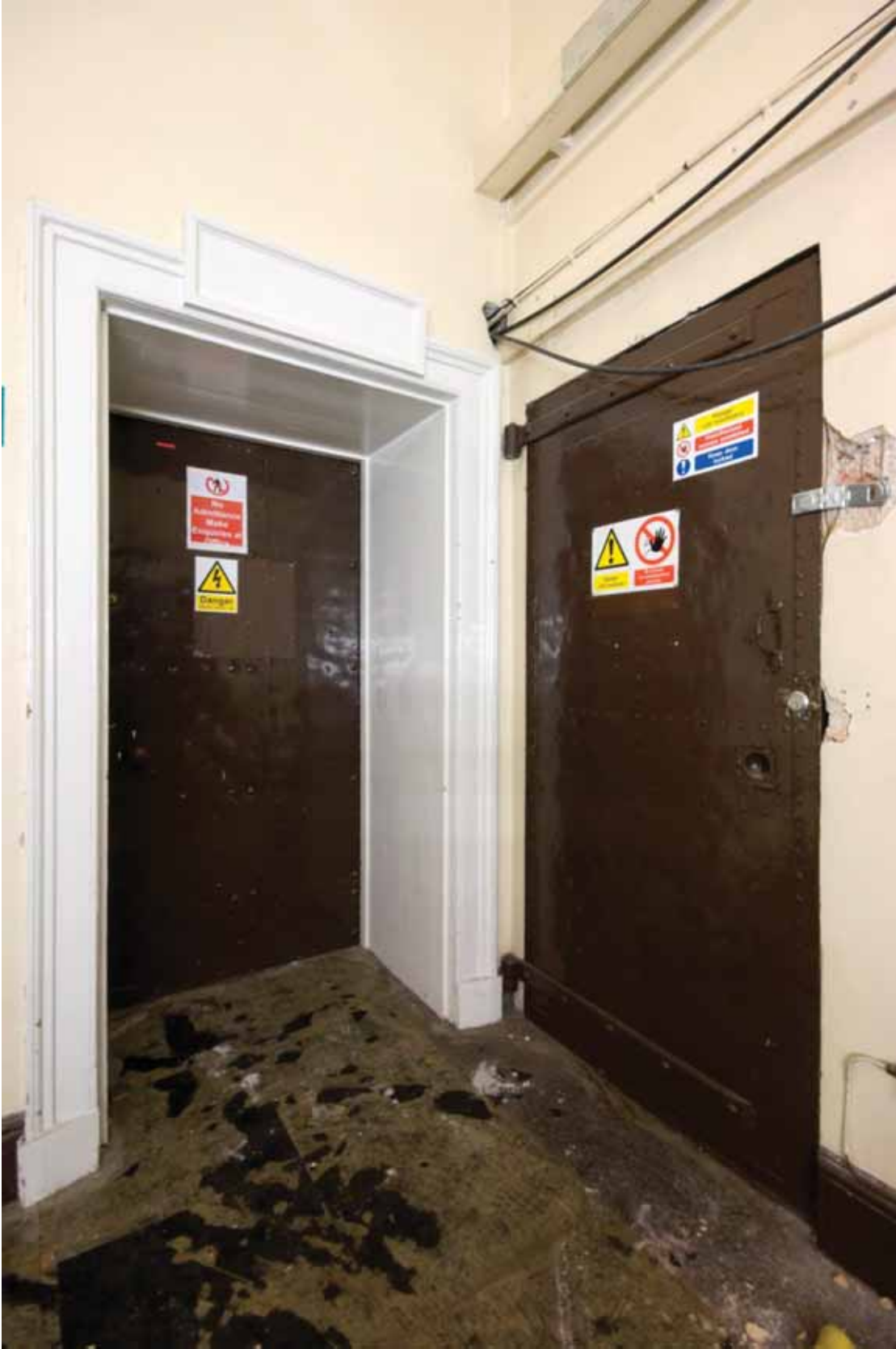
Plate 232: West (left) and north (right) walls of Corridor 04LG, looking north-west (EAF10 LG100 1072)
