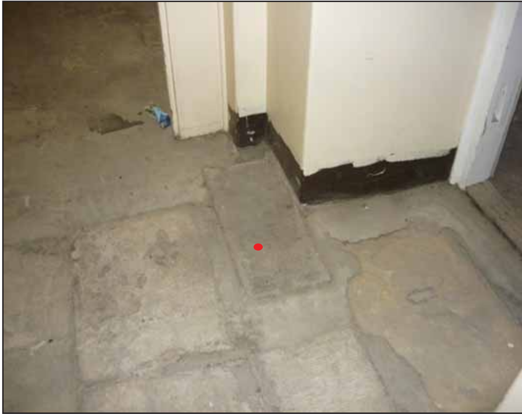
Plate 81: Floor in Corridor 1B with doorway into Room B51 (right) with cement base for World War Two shoring (red dot), looking north-west
