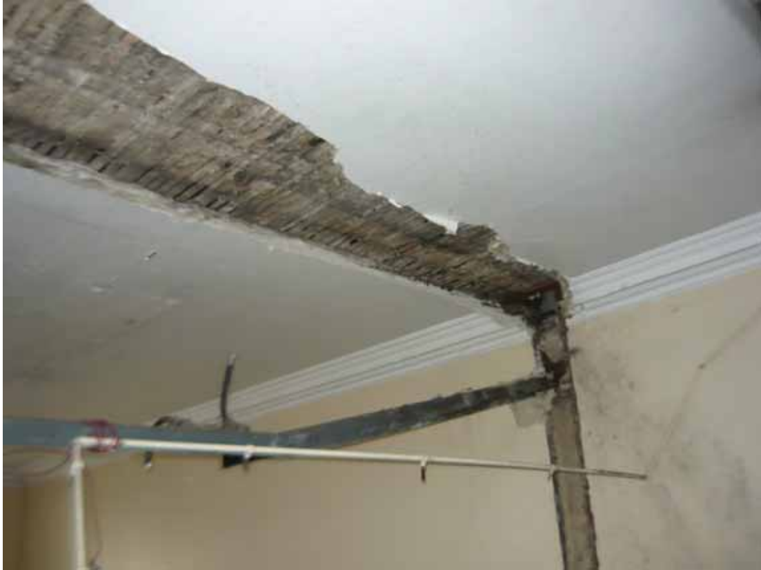
Plate 609: Scar of removed partition wall in Room S91, looking south-east (EAF10 BHD3 (49))
