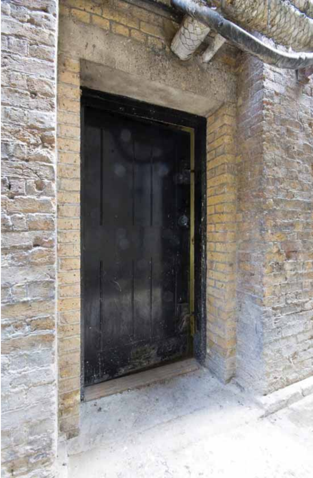
Plate 63: External doorway into Room B63 at the north end of the East Wing, looking south (DSC_1400_sitecode EAF10_© PCA Ltd 2010)
