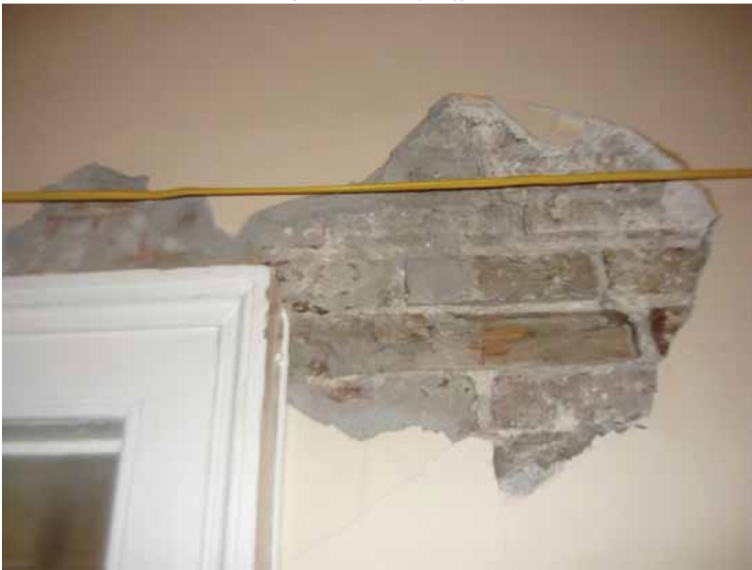
Plate 264: Timber lintel on the north side of the doorway in the west wall of Room M19, looking west (EAF10 BHD2 (105))
