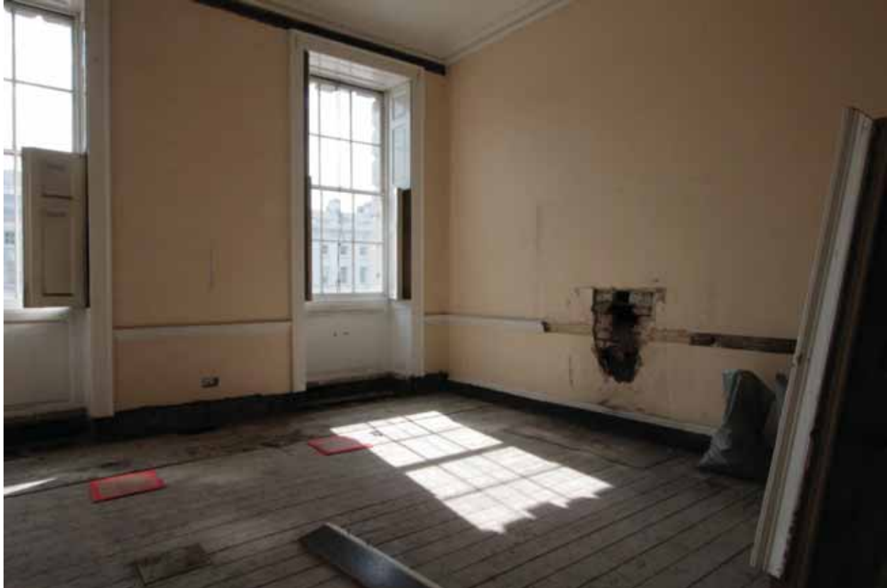
Plate 461: West (left) and north (right) walls in Room F01, looking north-west (EAF10 247)
