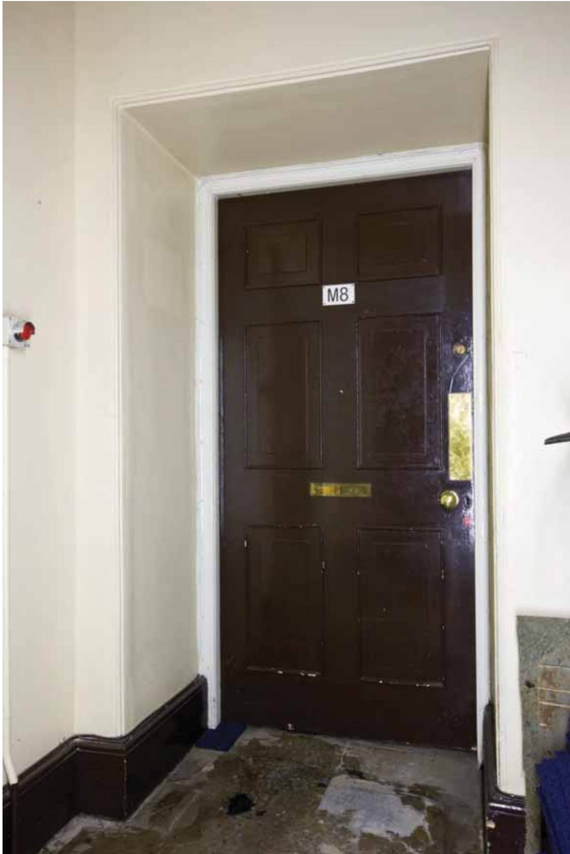
Plate 262: Doorway in the west wall of Corridor 07LG looking west (EAF10 LG100 0982)
