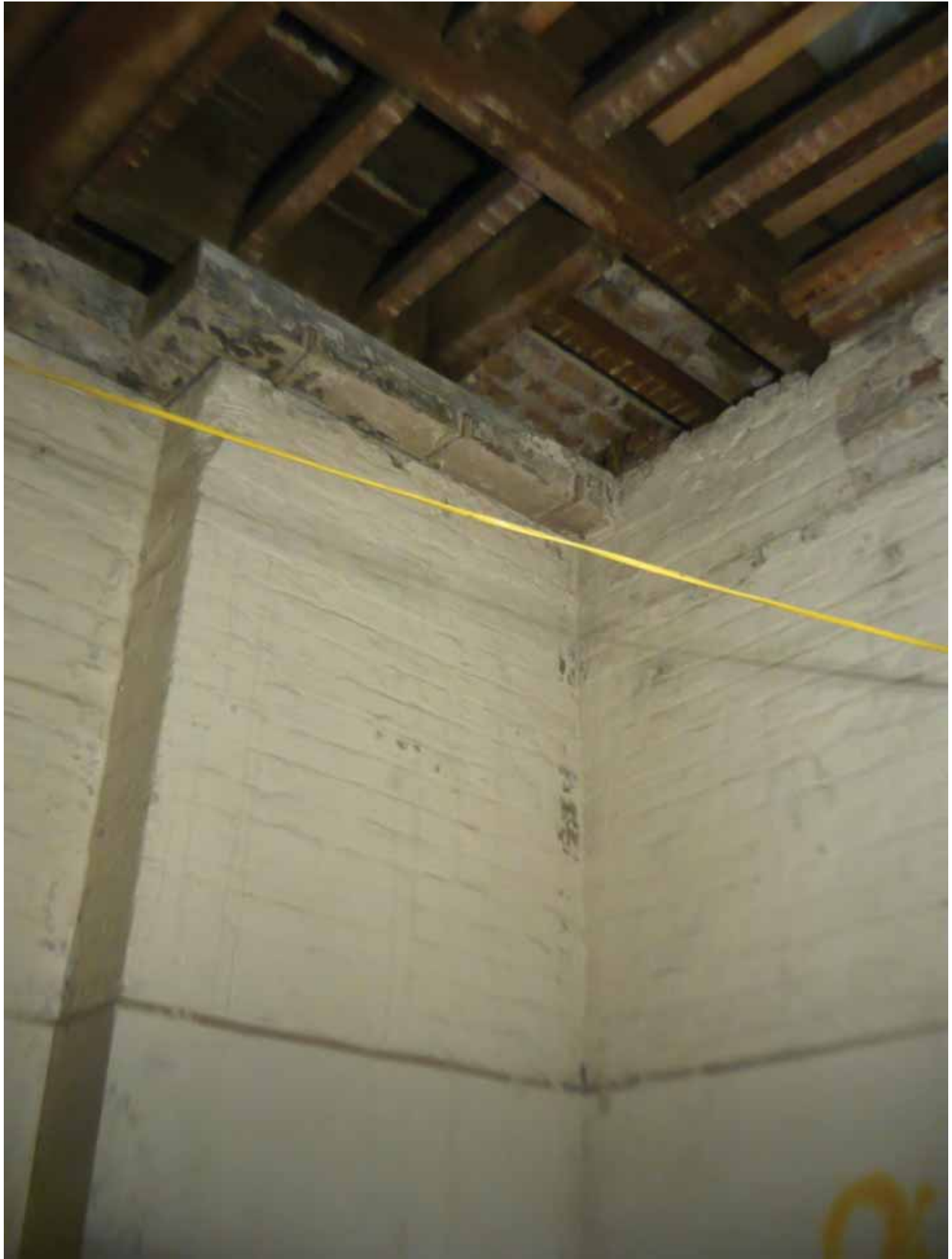
Plate 51: East (left) and south (right) walls in Room B48A, looking south-east (EAF10 BHD5 (20))
