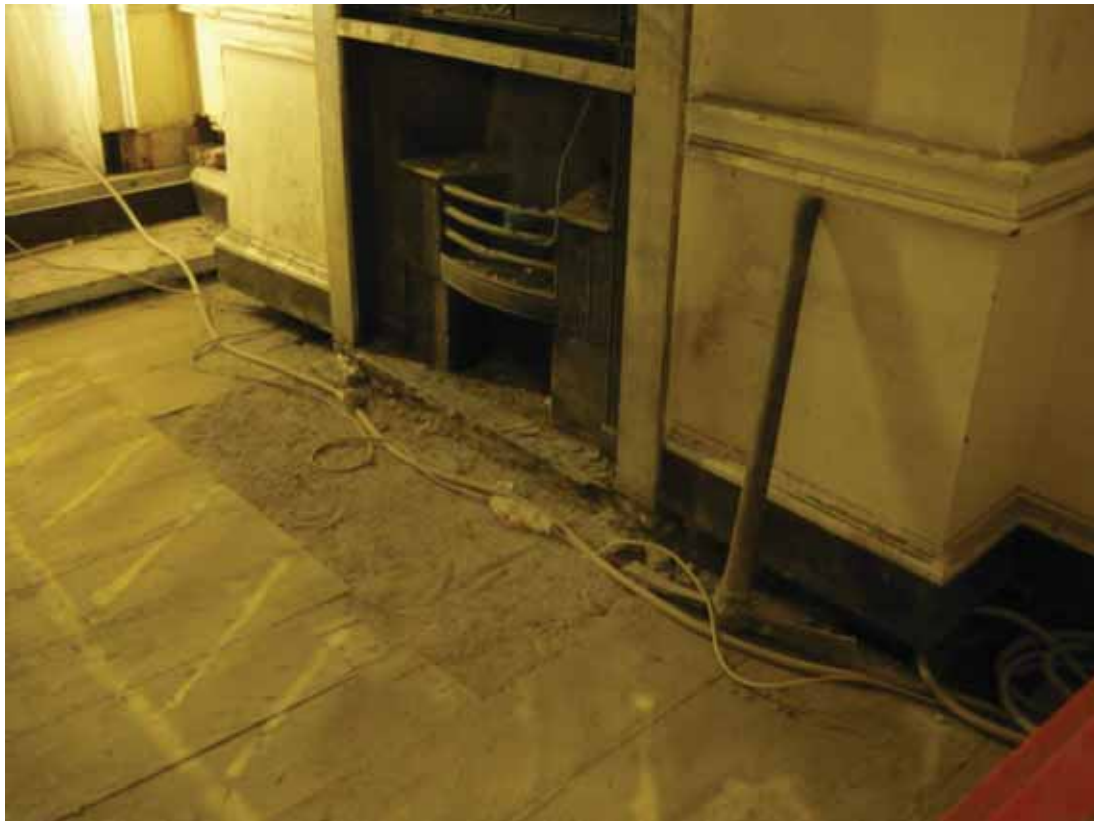
Plate 437: Fireplace in the south wall of Room G23, looking south-east (EAF10 BHD8 (118))
