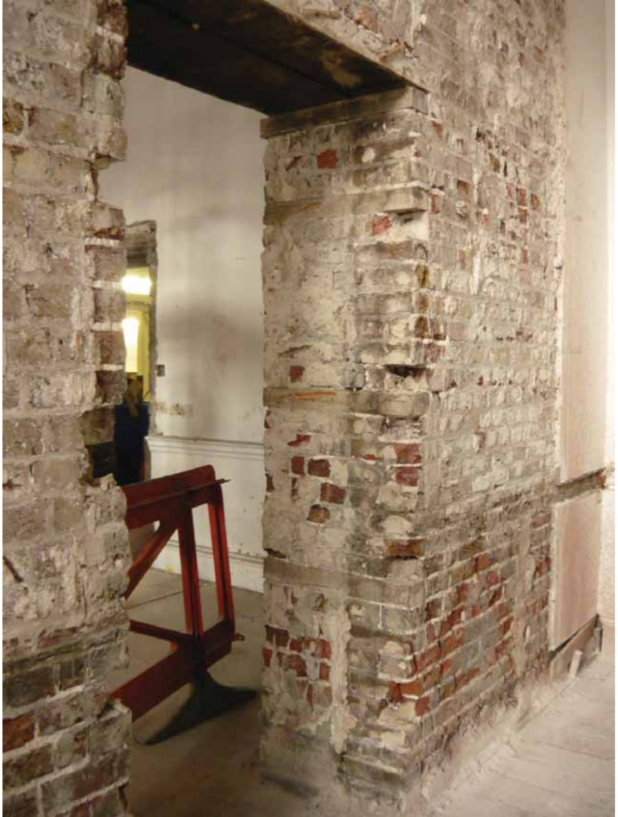
Plate 340: Doorway in the centre of the north wall in Room G41, looking north-east (EAF10 BHD8 (64))
