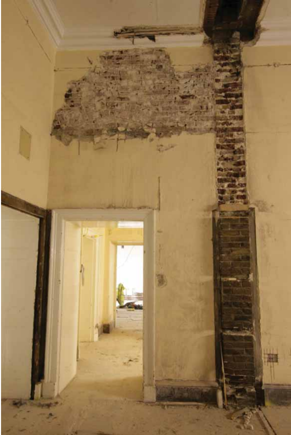
Plate 325: Doorway at the south end of the west wall in Room M29, looking west (EAF10 A100 051)
