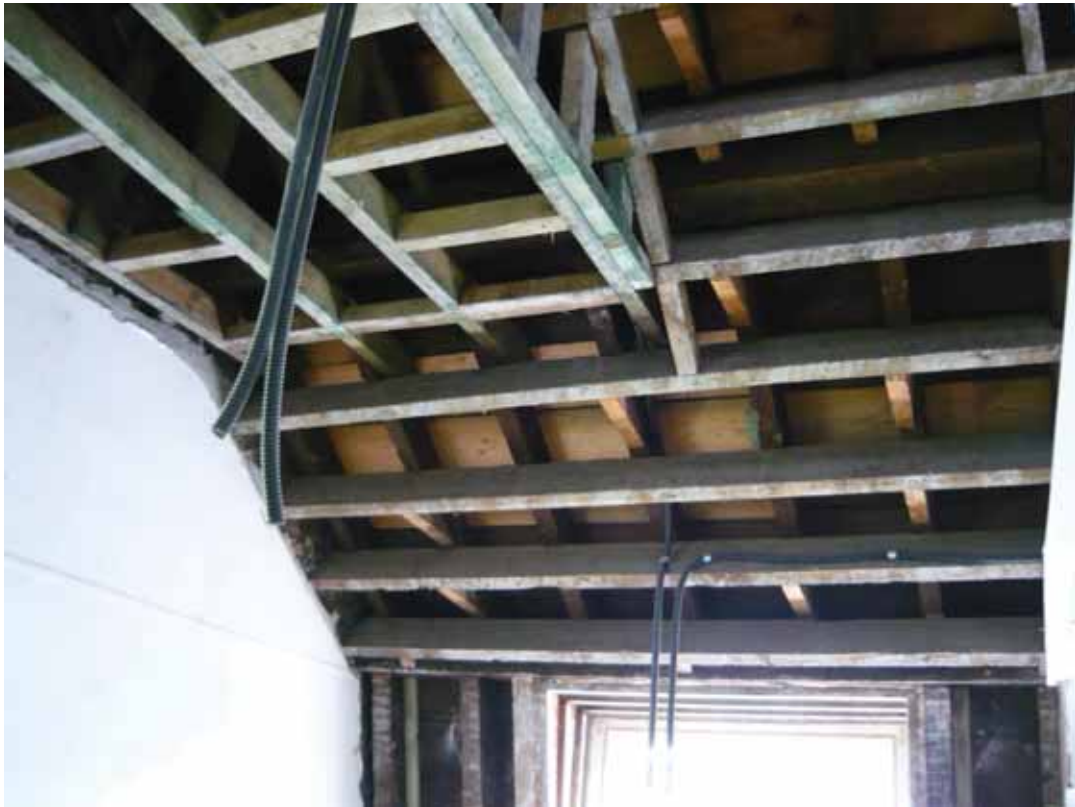
Plate 739: Roof structure above the east wall of Room T118, looking north-east (EAF10 BHD10 (31))
