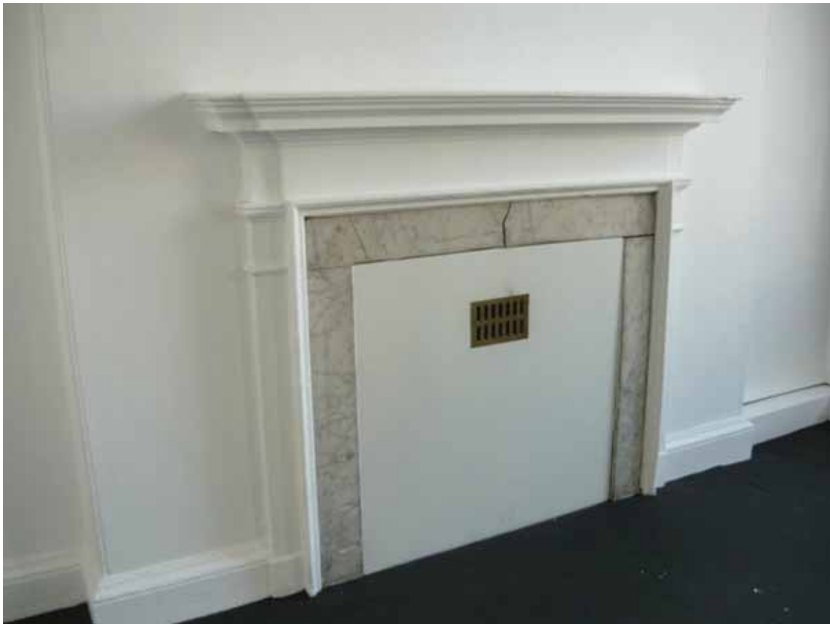
Plate 370: Fireplace (type 6) in the south wall of Room G08, looking south-west (EAF10 BHD1 (37))
