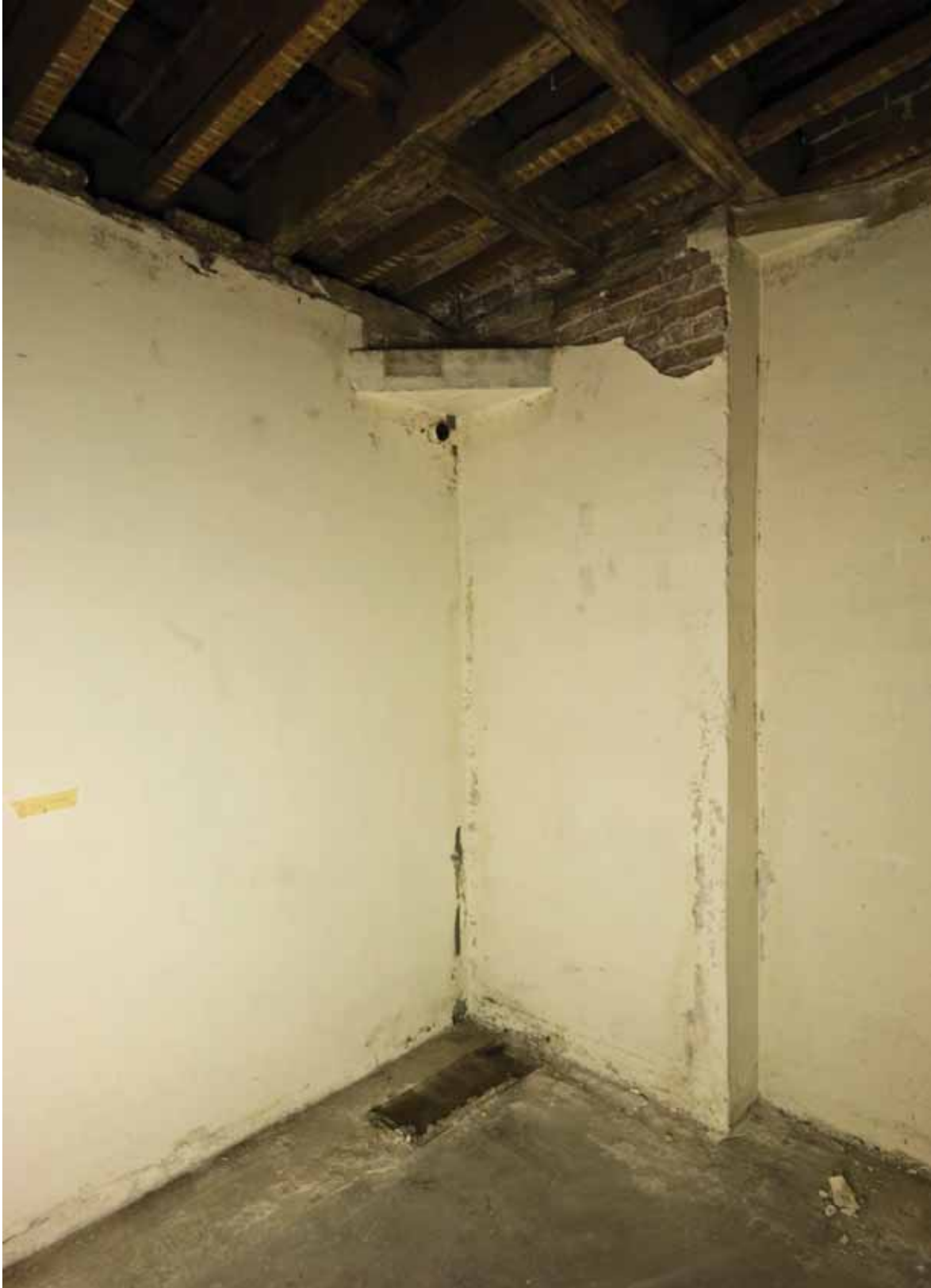
Plate 43a: East (left) and south (right) walls of Room B47C, looking south-east (DSC_1452 _sitecode EAF10_© PCA Ltd 2010)
