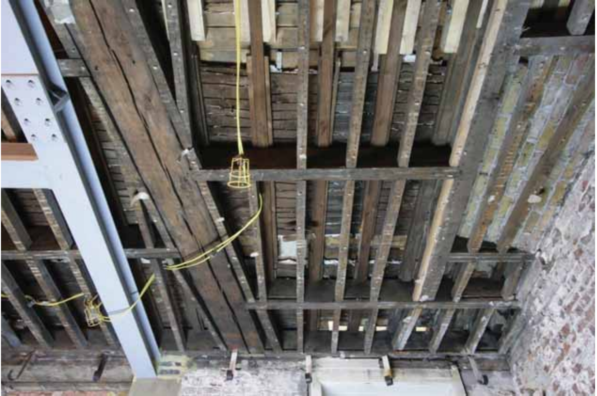
Plate 13: Primary and secondary floor joists visible following the removal of the lath and plaster ceiling in Room B43/B44, looking west (EAF10 A100 035)
