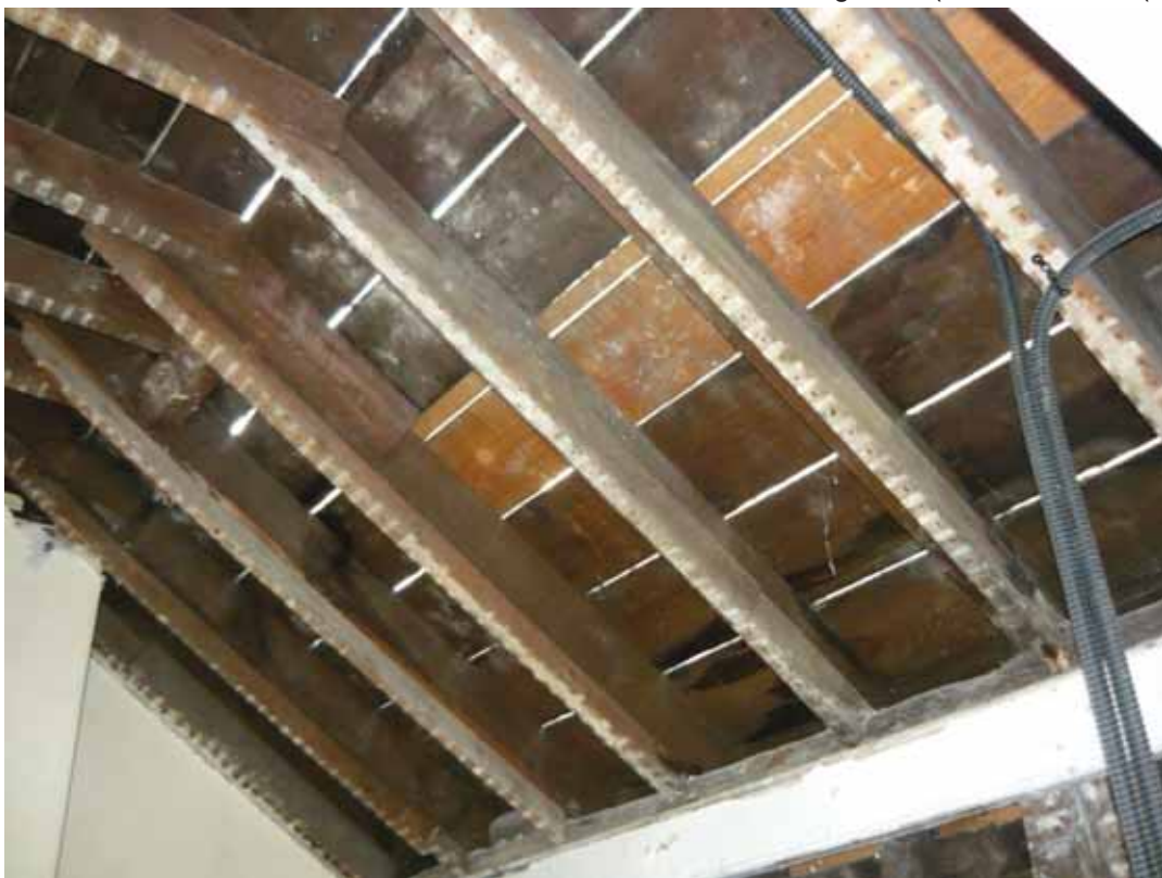
Plate 672: Common rafters above the west wall of Room T02, looking south-west (EAF10 BHD10 (57))
