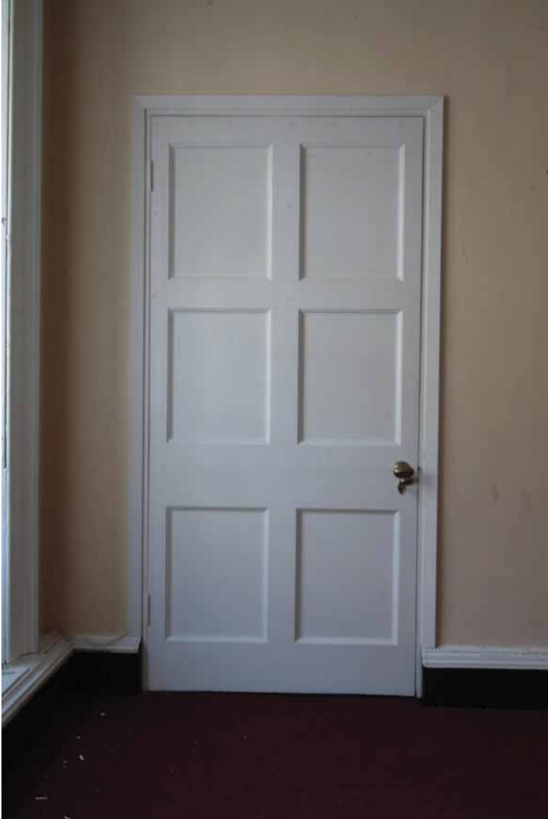
Plate 627: Doorway at the east end of the south wall in Room S17, looking south (EAF10 0141)
