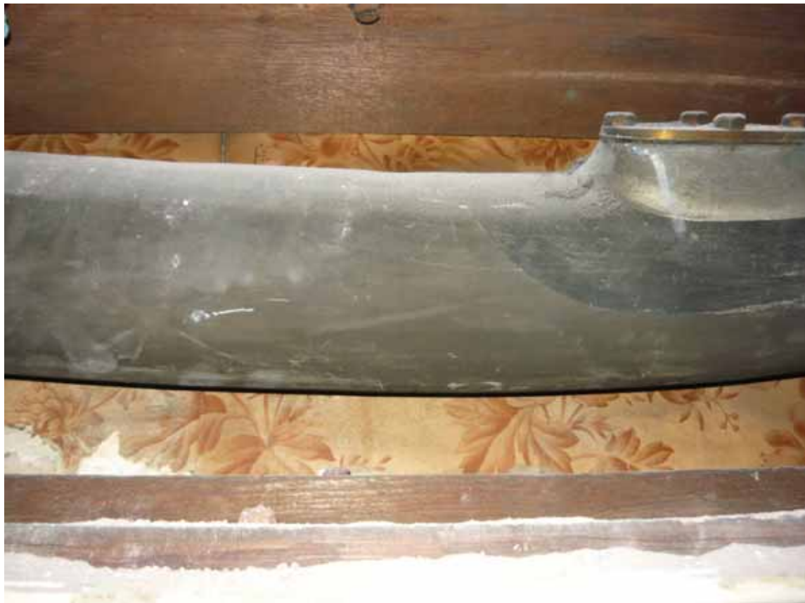
Plate 680: Lead pipe at the south end of Room T03, looking east (EAF10 BHD10 (61))
