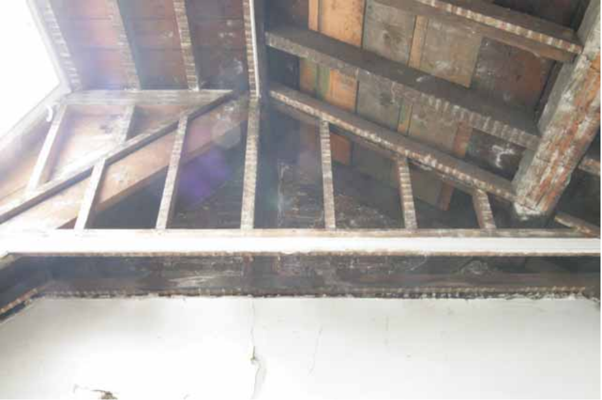
Plate 685: Dormer above the east wall and south wall of Room T05, looking south (EAF10 A100 013)
