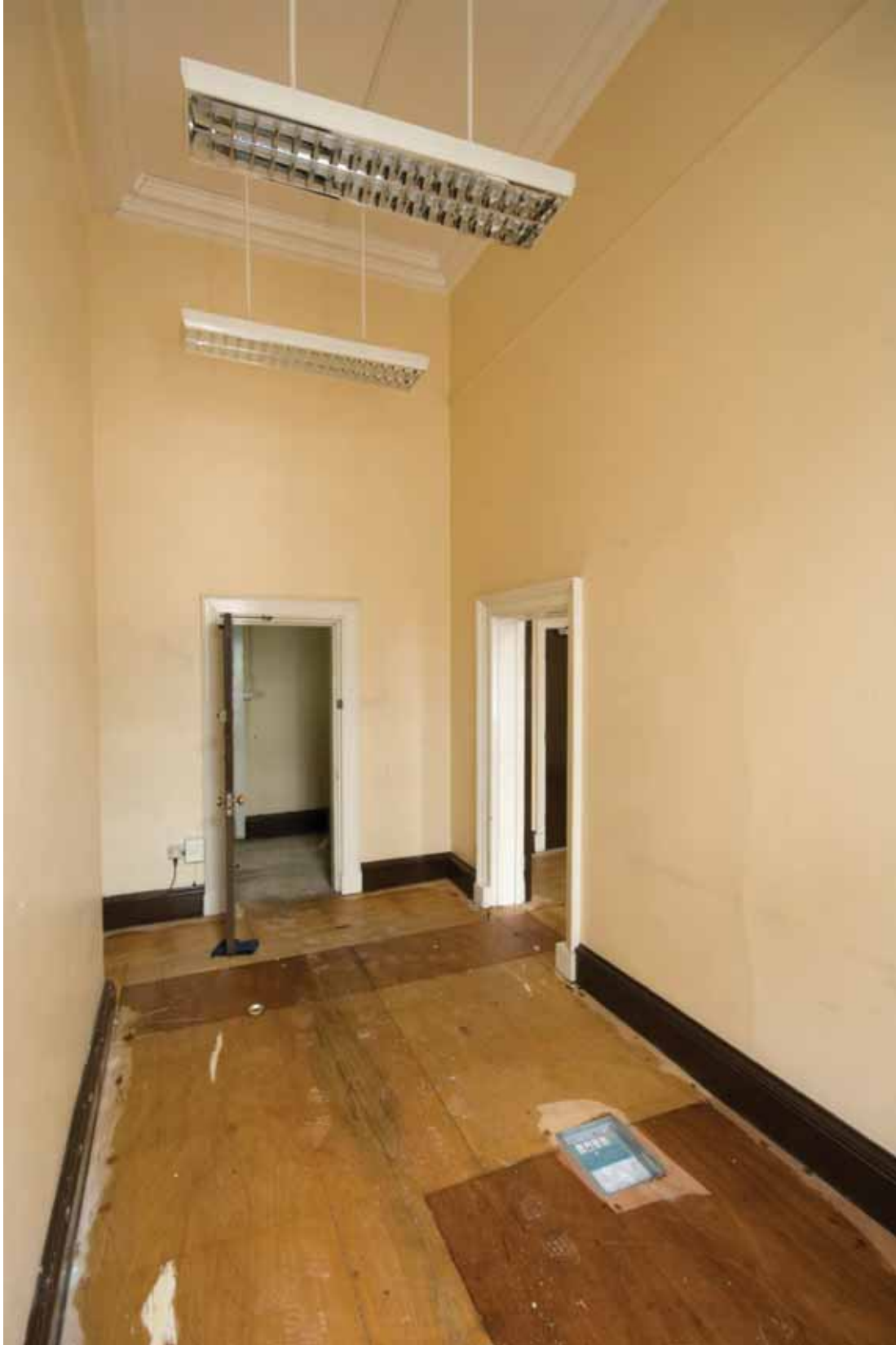
Plate 300: South (left), east (centre) and north (right) walls in Room M27, looking west (EAF10 LG100 1007)
