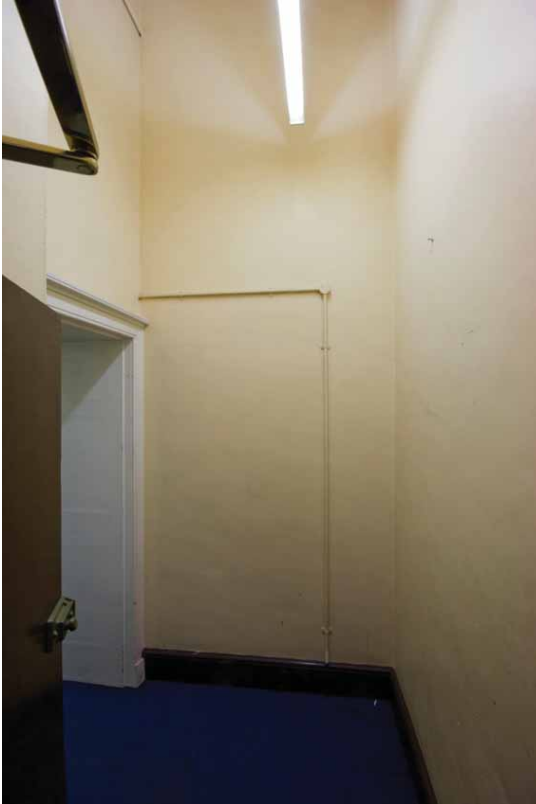
Plate 201: East (left), south (centre) and west (right) wall of added passage in Room M16, looking south (EAF10 LG100 1095)
