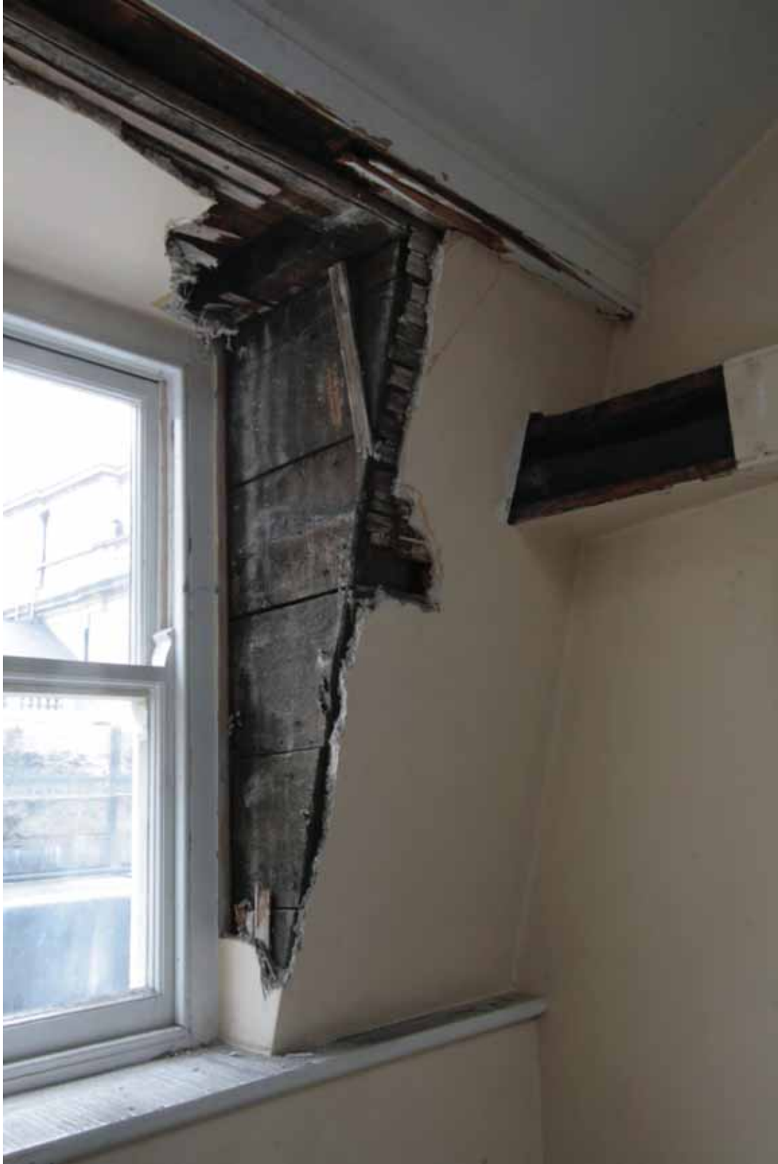
Plate 782: East (left) and south (right) walls in Room T25, looking south-east (EAF10 191)
