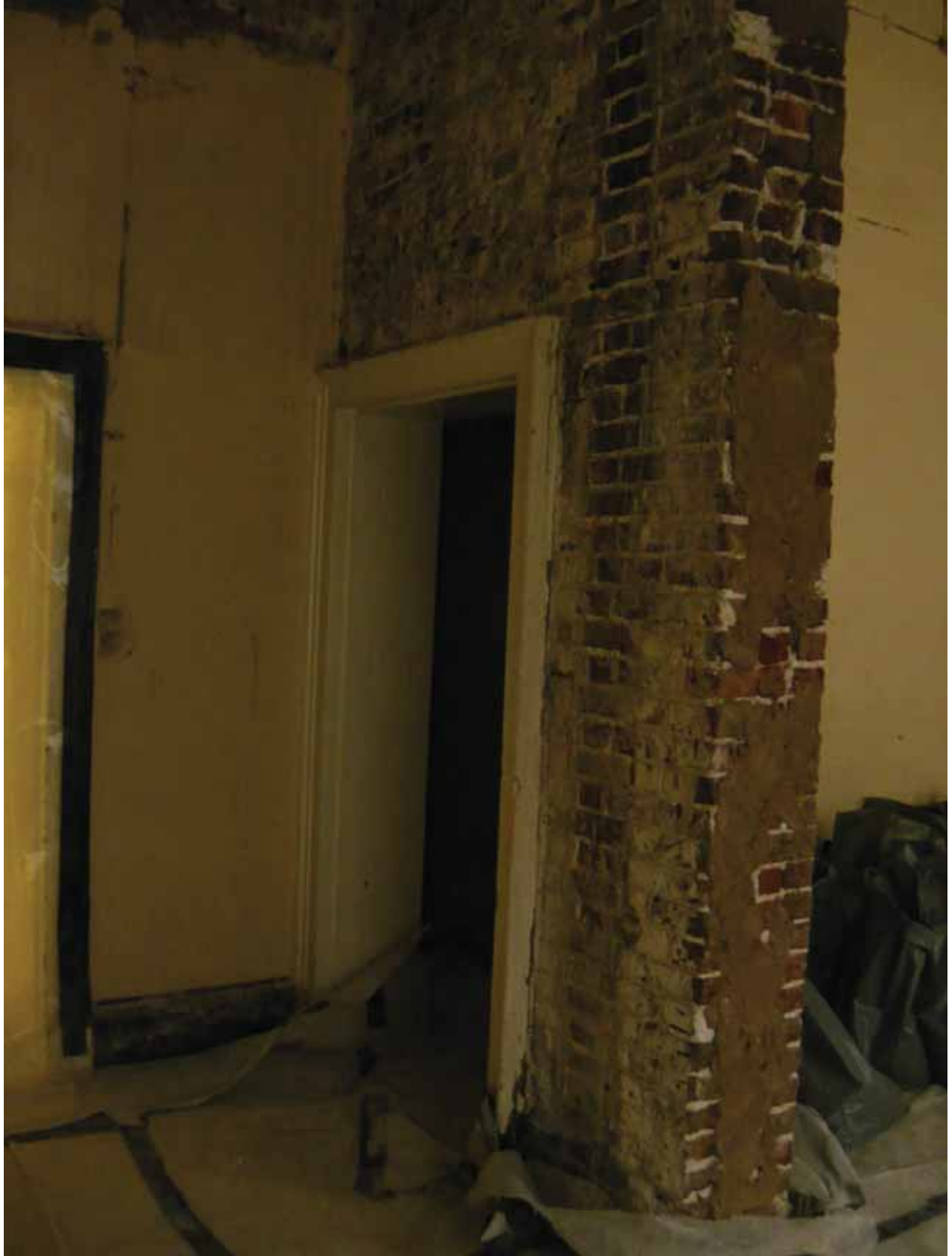
Plate 322: West end of north partition wall in Room M29b, looking north-west (EAF10 BHD6 (17))
