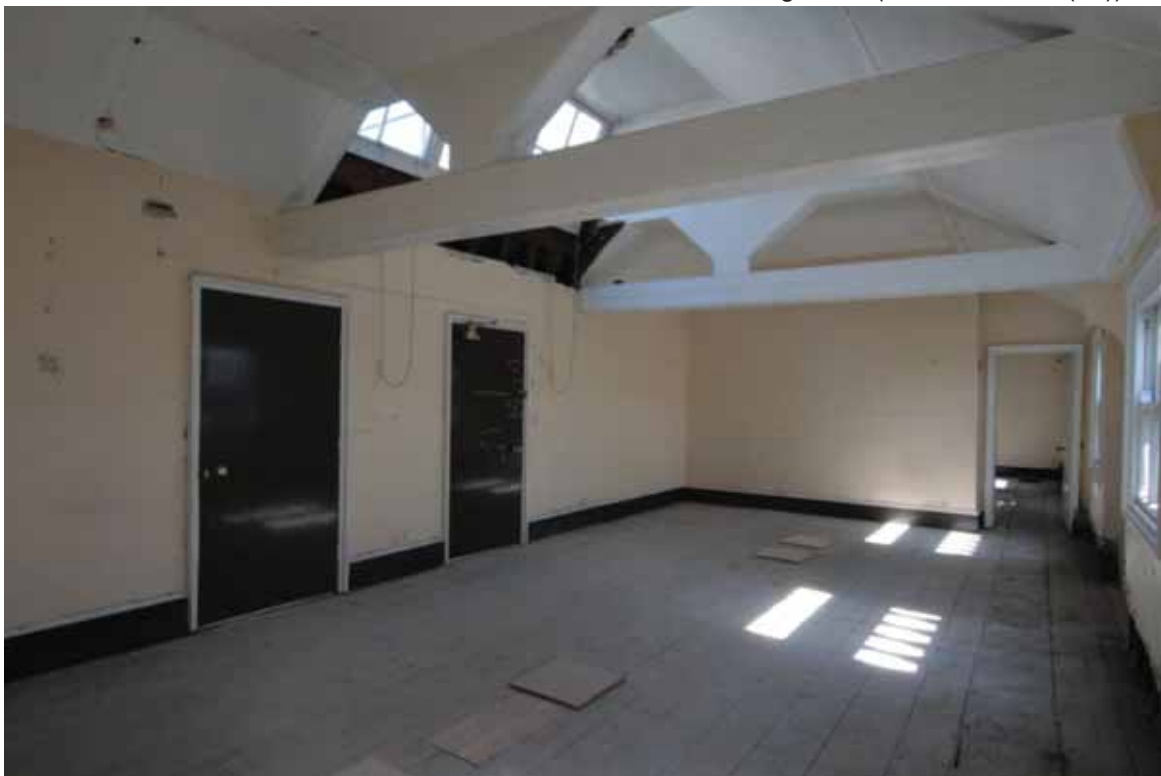
Plate 666: East (left) and south (right) walls of Room T02, looking south-east (EAF10 204a)
