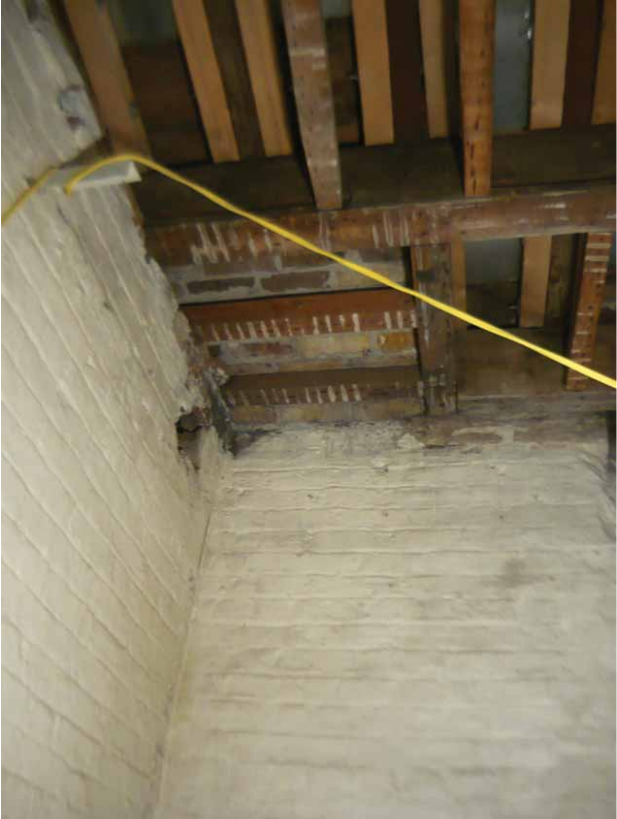
Plate 52: North (left) and west (right) walls in Room B48B, looking north-east (EAF10 BHD5 (29))
