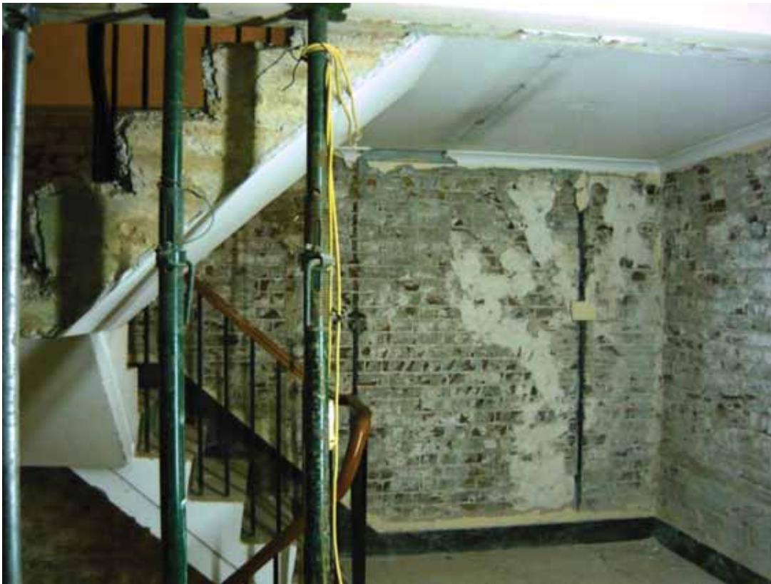
Plate 250: North (left and centre) and east (right) walls (upper level) in Corridor 06LG looking north (EAF10 BHD7 (11))
