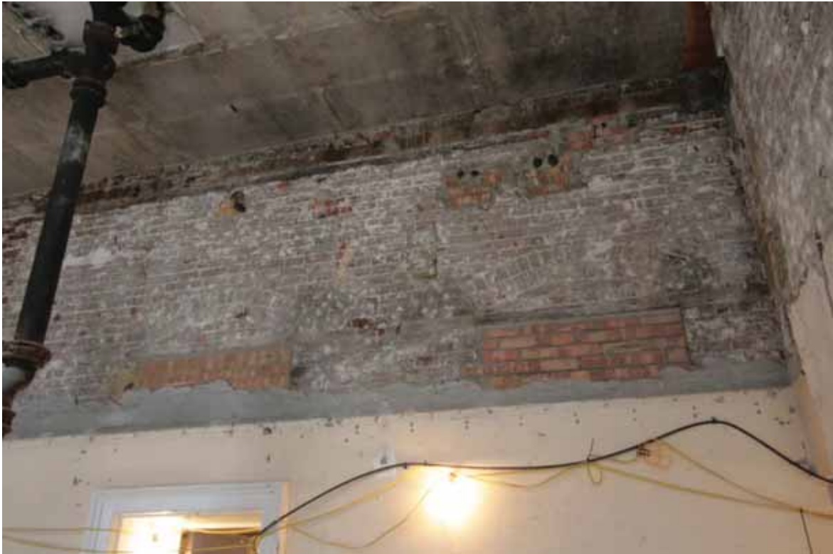
Plate 287: North end of the upper part of the west wall in Room M116, looking west (EAF10 293a)
