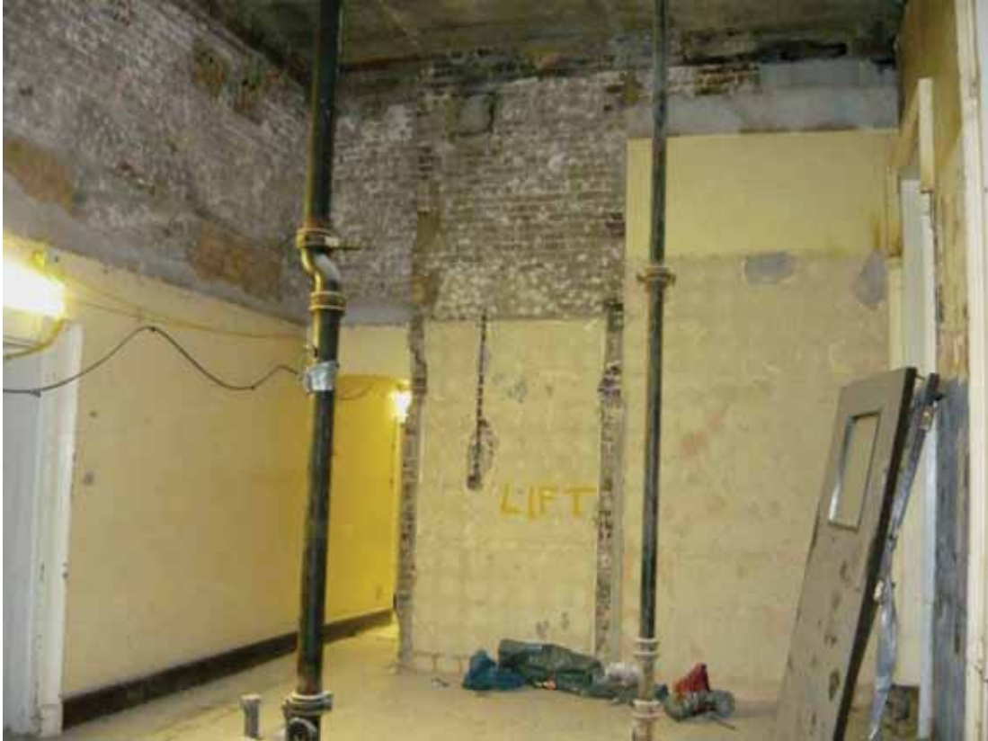
Plate 283: West (left) and north (centre and right) walls of Room M116, looking north (EAF10 BHD6 (79))
