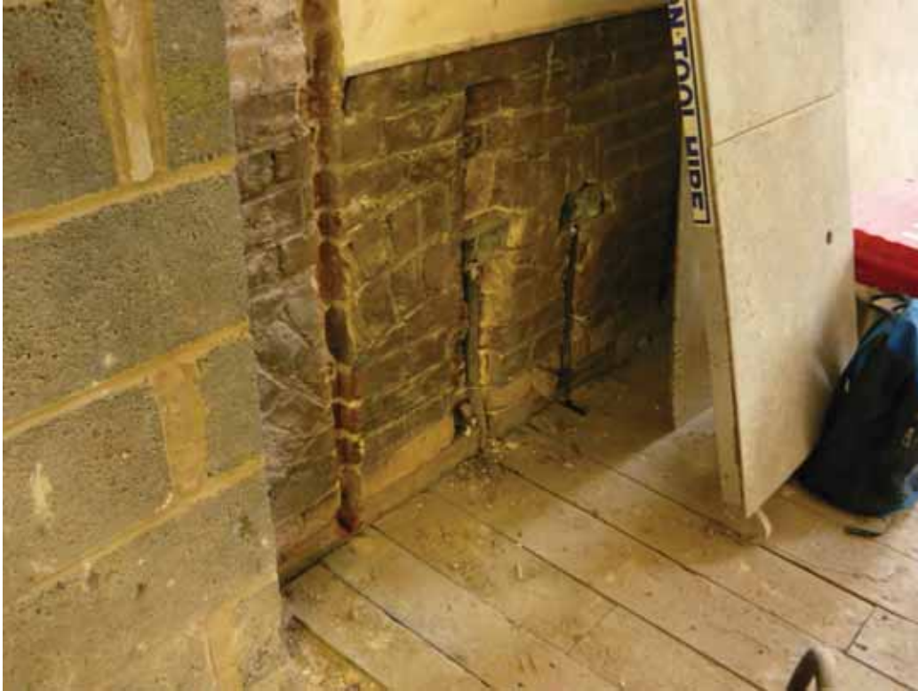
Plate 464c: Brick arch to the east of the fireplace in the south wall of Room F02, looking south (EAF10 BHD8 (147))
