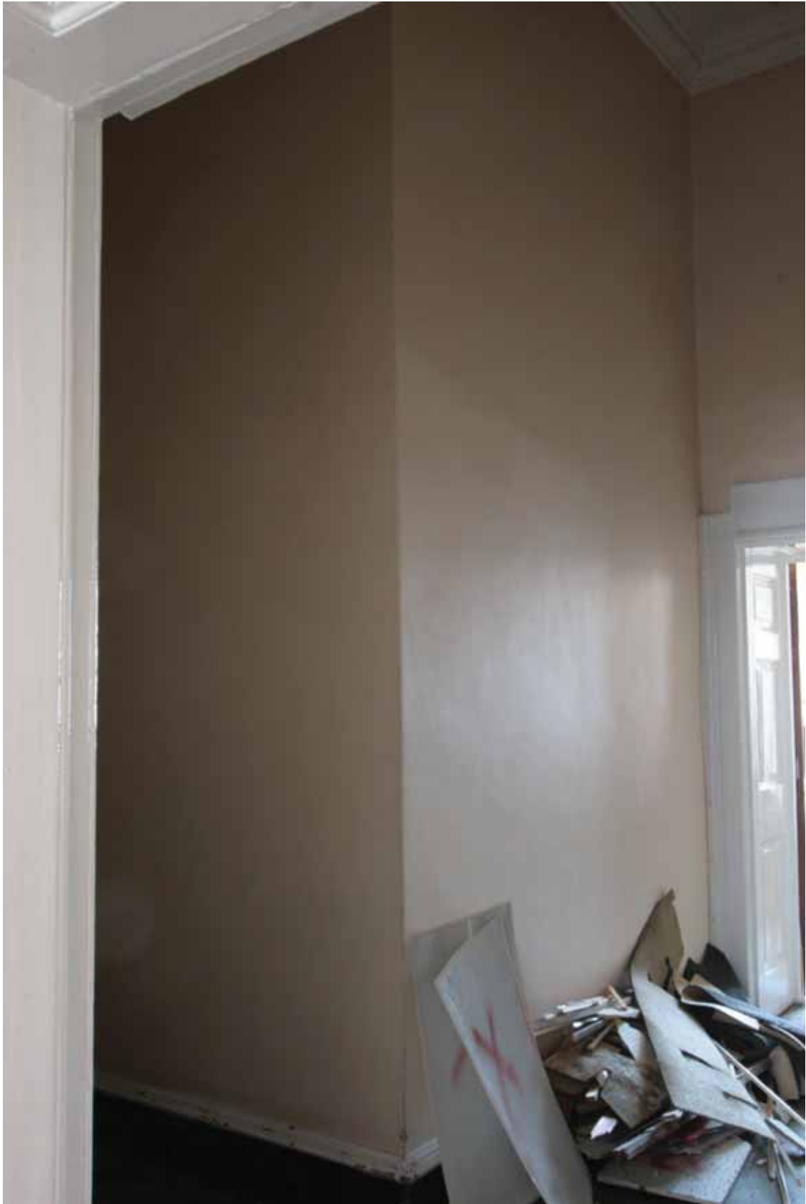
Plate 506: North-east corner of the dumb waiter in Corridor 07F, looking south-west (EAF10 172)
