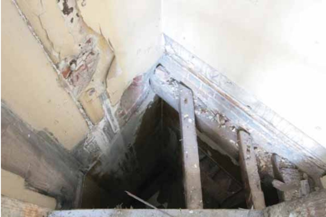
Plate 356: Inside cupboard at the south end of the east wall in Room G03, looking down and east (EAF10 274A)
