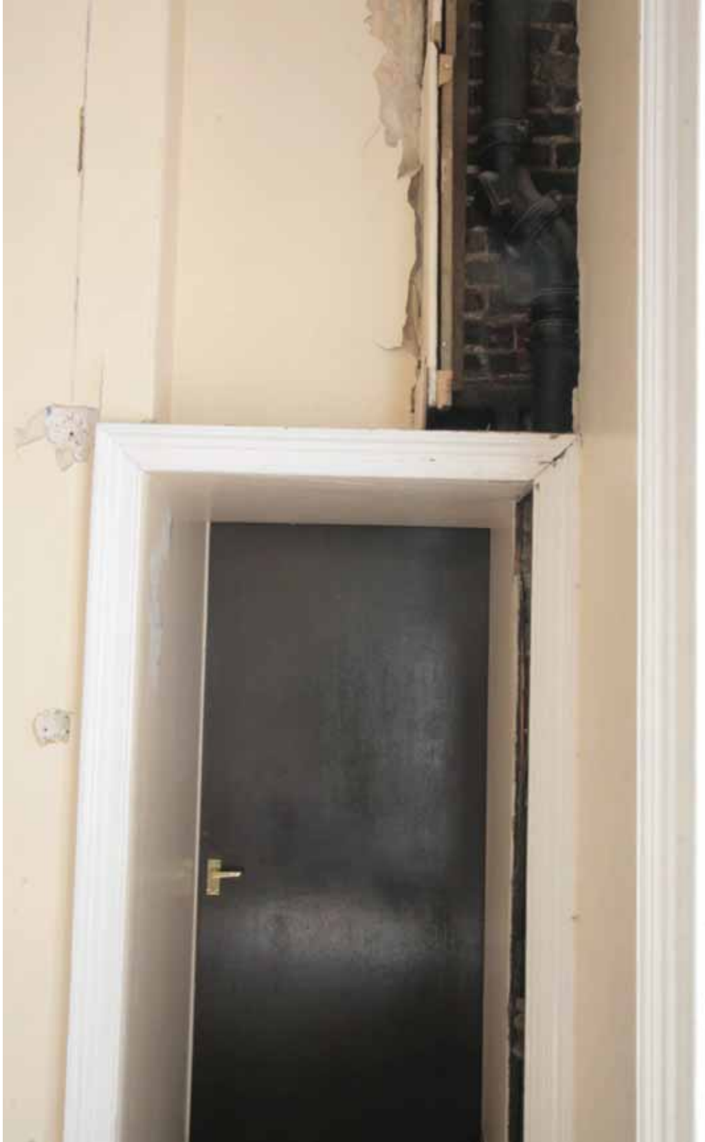
Plate 179: Doorway at the west end of the south wall in Room M09, looking south (EAF10 305)
