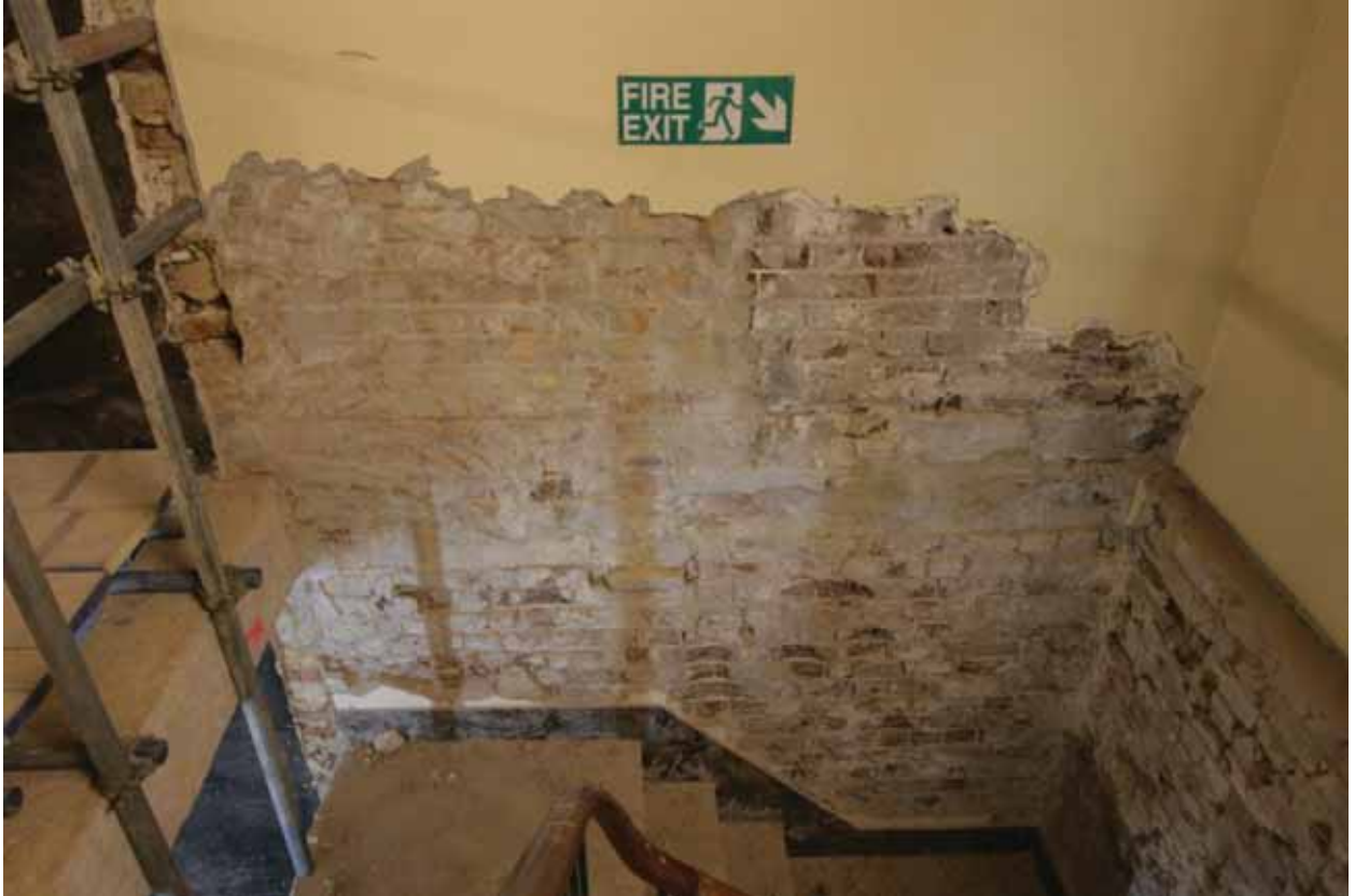
Plate 393: North end of the west wall of Corridor 08G, looking west (EAF10 A100 025)
