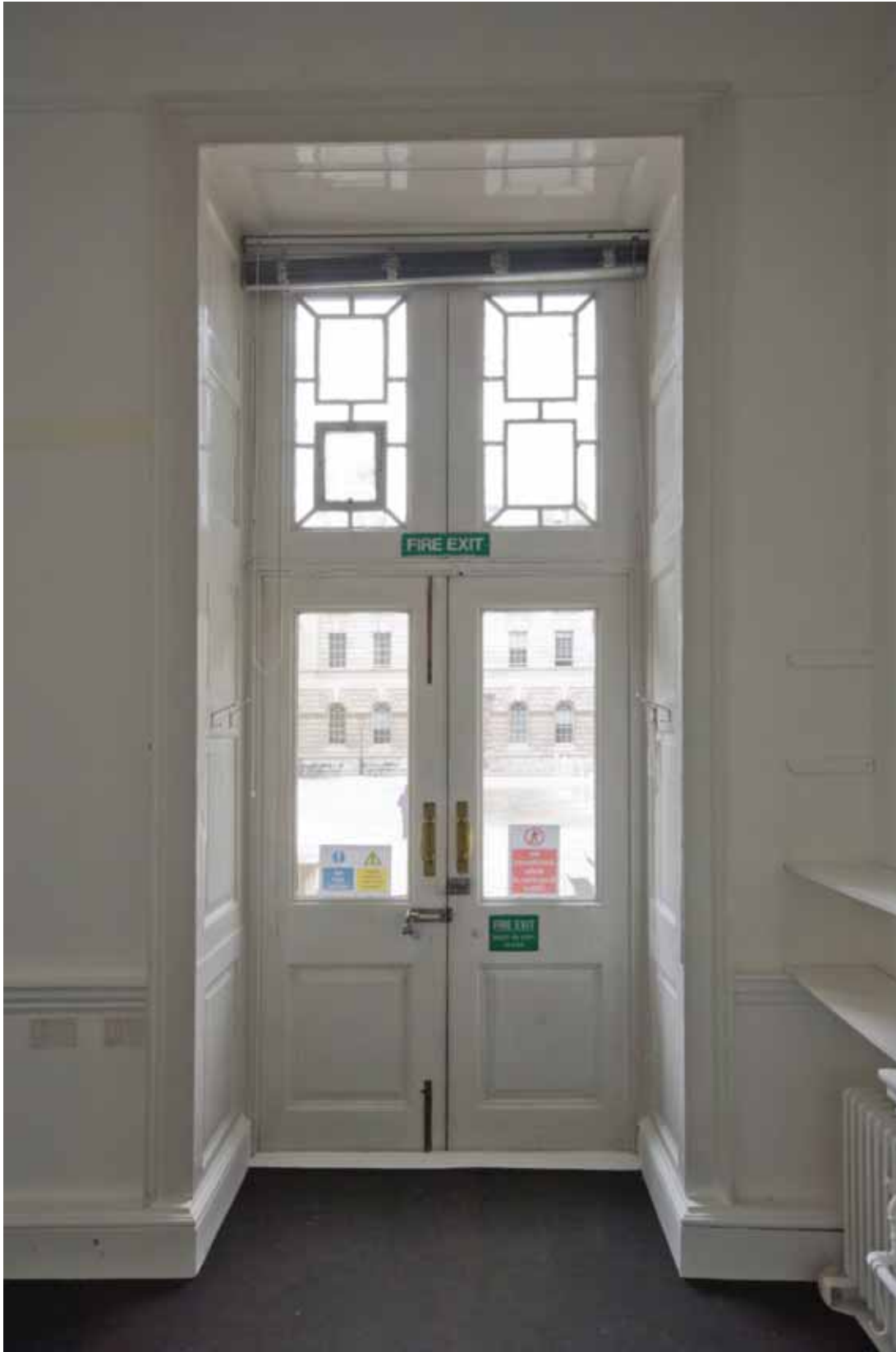
Plate 344: Doorway (type 37) at the north end of the west wall in Room G01, looking west (DSC_0836 sitecode EAF10 © PCA Ltd 2010)
