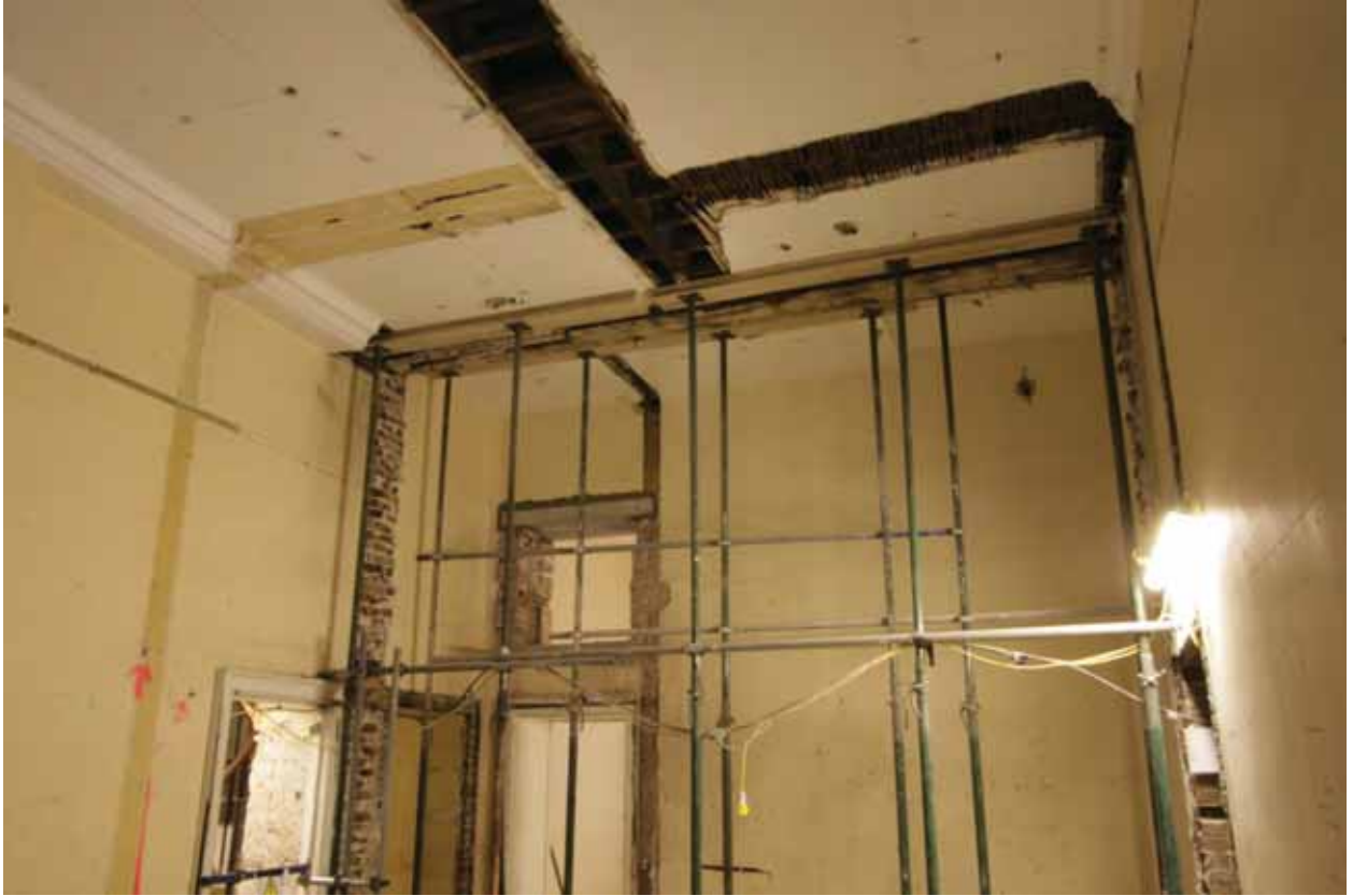
Plate 303: Scars of removed partition walls in Room M26/M27, looking south-west (EAF10 A100 033)
