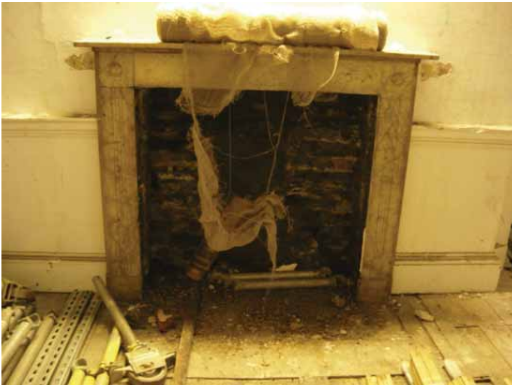
Plate 413: Fireplace (type 21) in the north wall of Room G17, looking north (EAF10 BHD8 (119))
