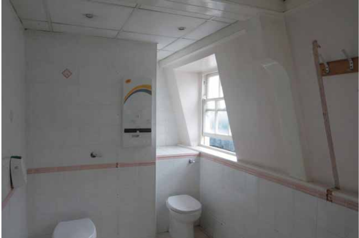
Plate 757: North partition (left) and east (right) walls in Room T20, looking north-east (EAF10 42)
