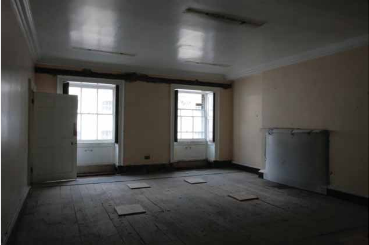
Plate 624: North (left), east (centre) and south (right) walls in Room S16, looking south-east (EAF10 234)
