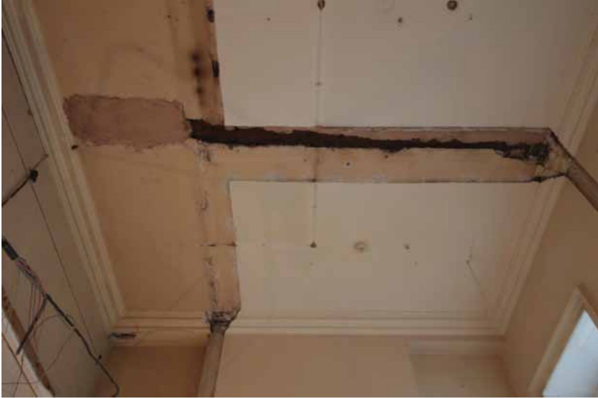
Plate 330: Scars of removed partition walls on the ceiling of Room M117, looking north (EAF10 301)
