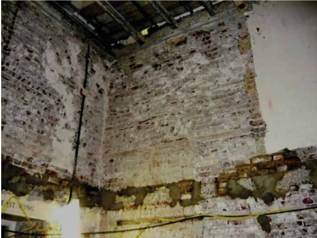
Plate 256: North (left) and east (right) walls of Corridor 06LG looking north-east (EAF10 BHD8 (104))
