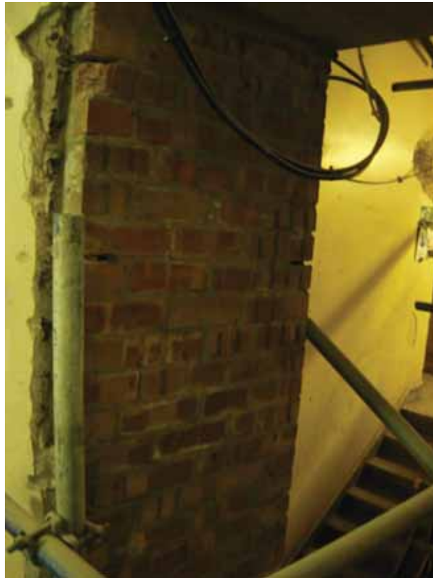
Plate 235: East reveal of the south doorway in Corridor 04LG, looking south-east (EAF10 BHD8 (141))
