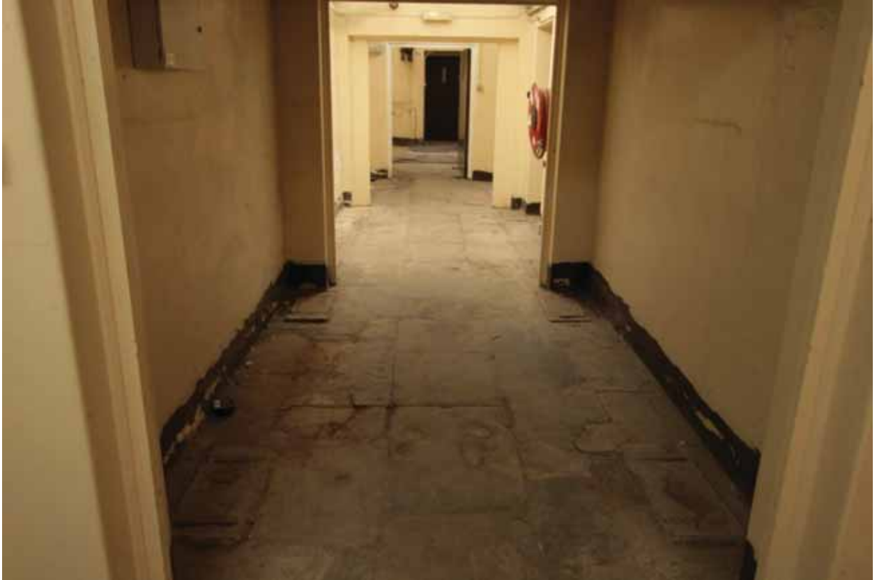
Plate 83: View north from Corridor 1D to Corridors 1C, 1B and 1A and Stairs 01 (EAF10 D100 024)
