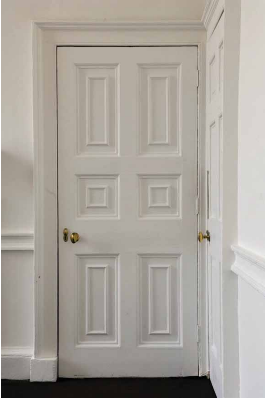
Plate 363: Door at the east end of the north wall in Room G05, looking north (EAF10 B100 0915)
