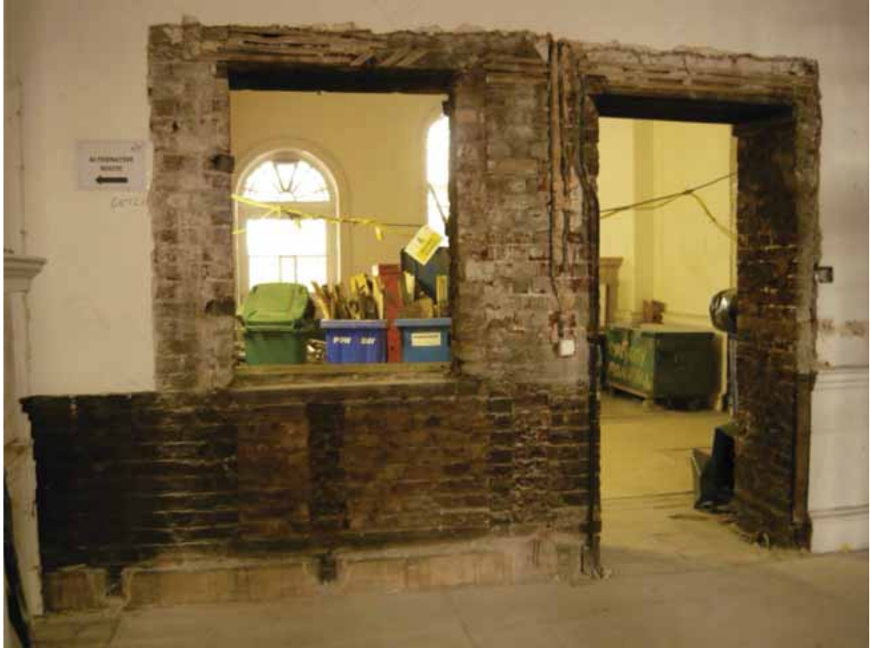
Plate 347: Doorway and internal window opening in the east wall of Room G01, looking east (EAF10 BHD8 (70))
