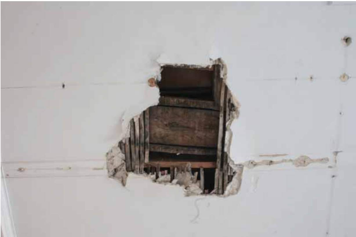
Plate 453: East-west principal floor joist revealed when east-west partition in Room F68 was removed looking north-east (EAF10 249)
