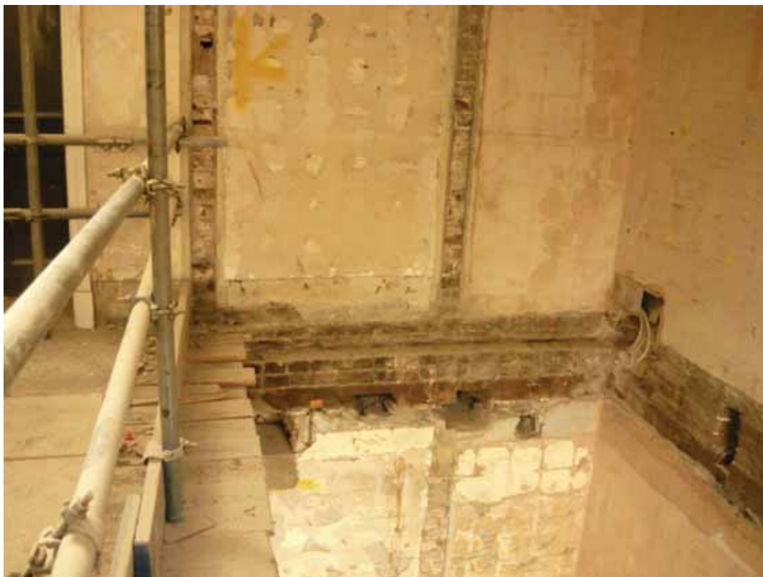
Plate 763: West (left) and north (right) walls in Room T20, looking west (EAF10 BHD8 (96))
