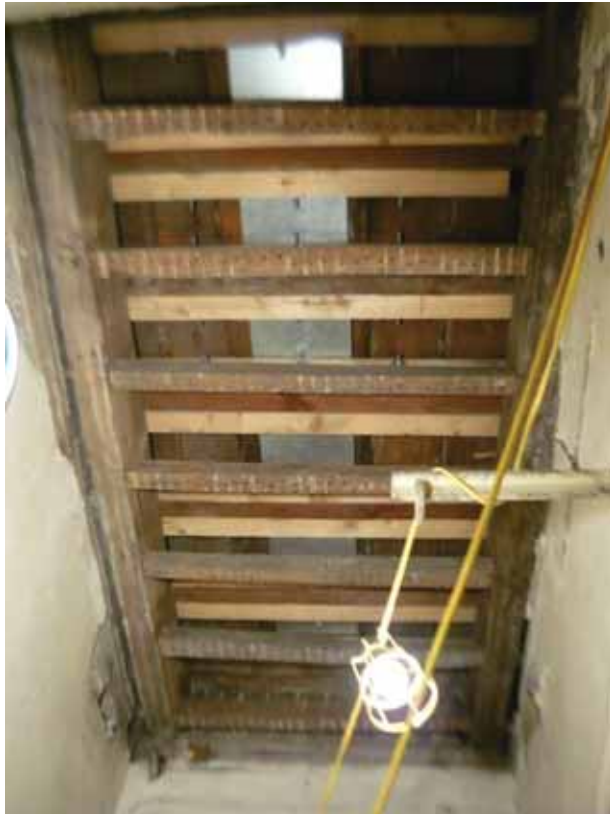
Plate 50: Primary and secondary floor joists exposed above Room B48D, looking south (EAF10 BHD5 (47))
