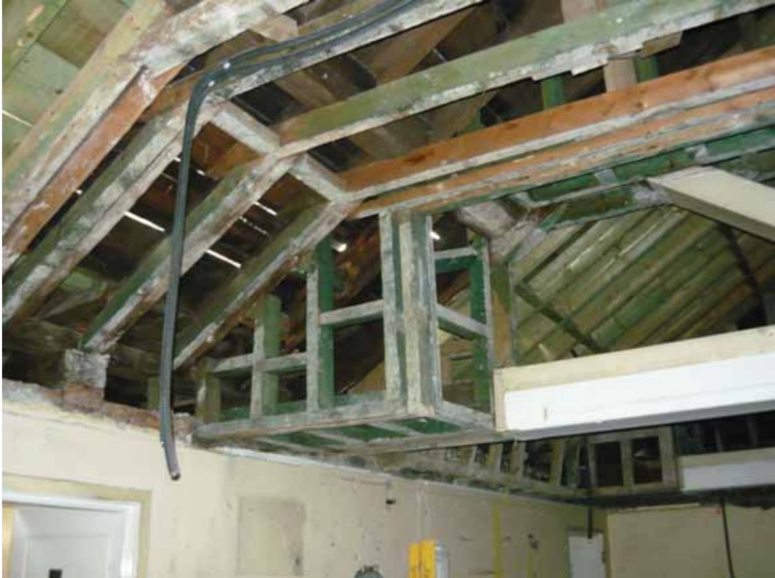
Plate 654: Roof structure above the east wall of Room T120, looking south-east (EAF10 BHD10 (49))
