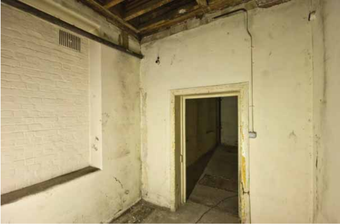
Plate 32: West (left) and north (right) walls of Room B47C, looking north-west (DSC_1457 _sitecode EAF10 © PCA Ltd 2010)
