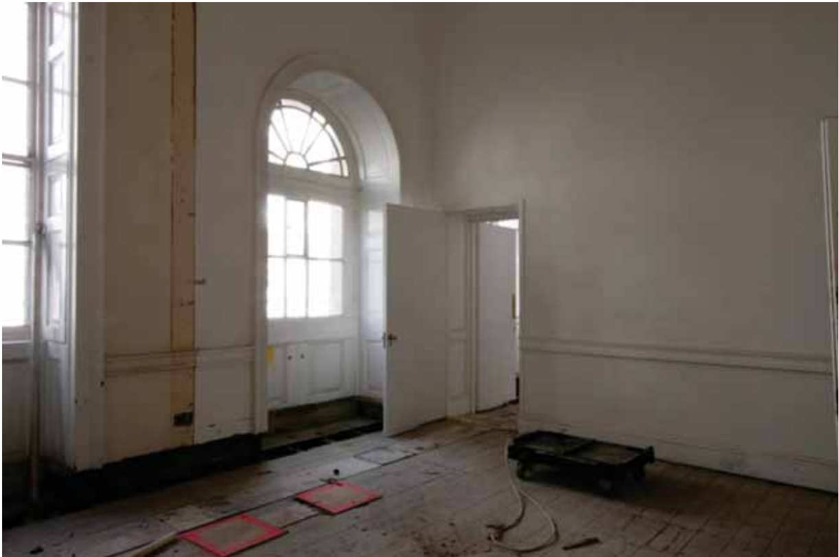
Plate 418: East (left) and south (right) walls in Room G18, looking south-west (EAF10 B100 0885)
