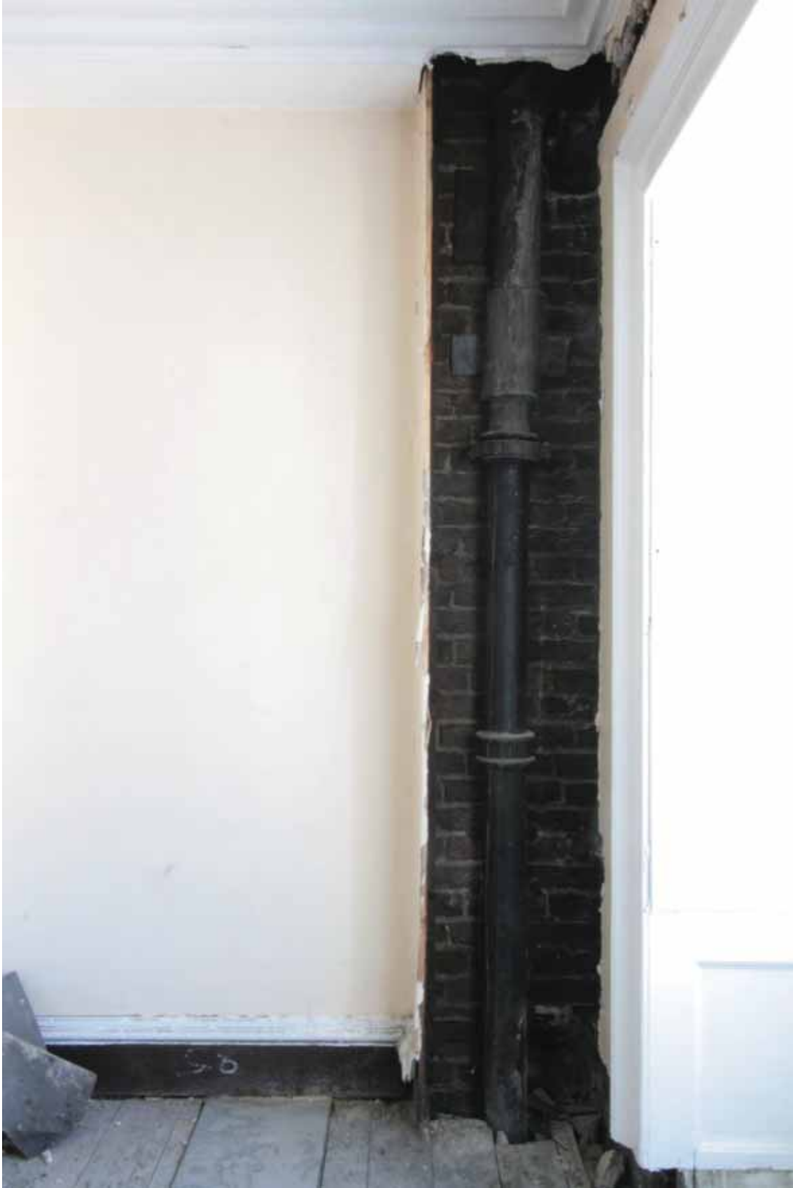
Plate 573: Boxed in pipe in the south-west corner of Room S08, looking south (EAF10 223)
