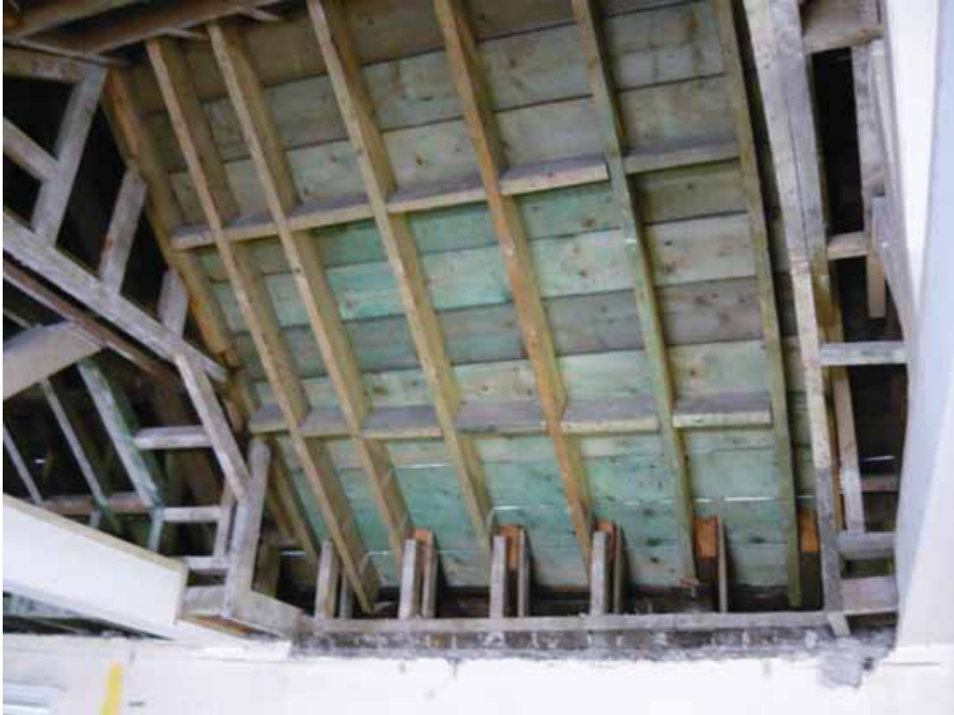
Plate 736: Roof structure above the centre (between the two trusses) of the west wall in Room T117, looking west (EAF10 BHD10 (36))
