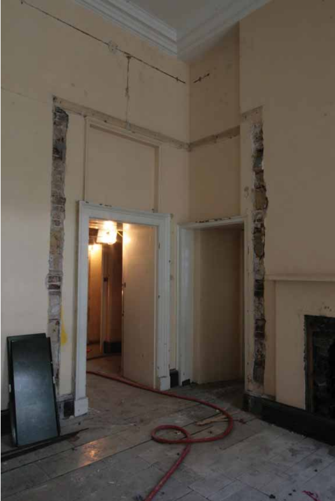
Plate 323: West (left) and north (right) walls in Room M29a, looking north-west (EAF10 300)
