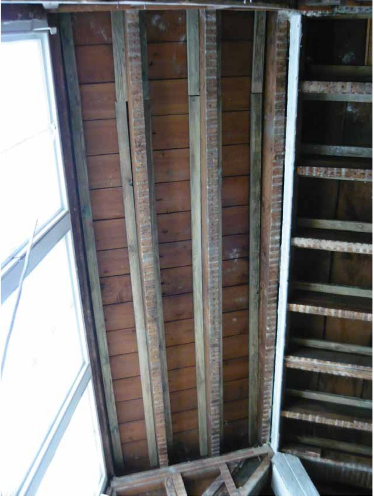
Plate 765: Dormer window in the west side of the roof above Room T22, looking north (EAF10 BHD10 (21))
