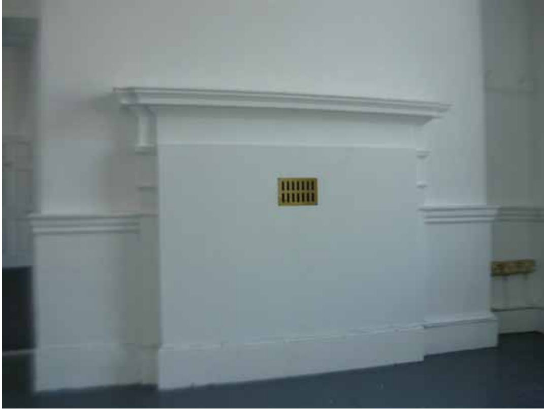
Plate 338: Fireplace (type 6) in the south wall of Room G41, looking south-east (EAF10 BHD1 (61))
