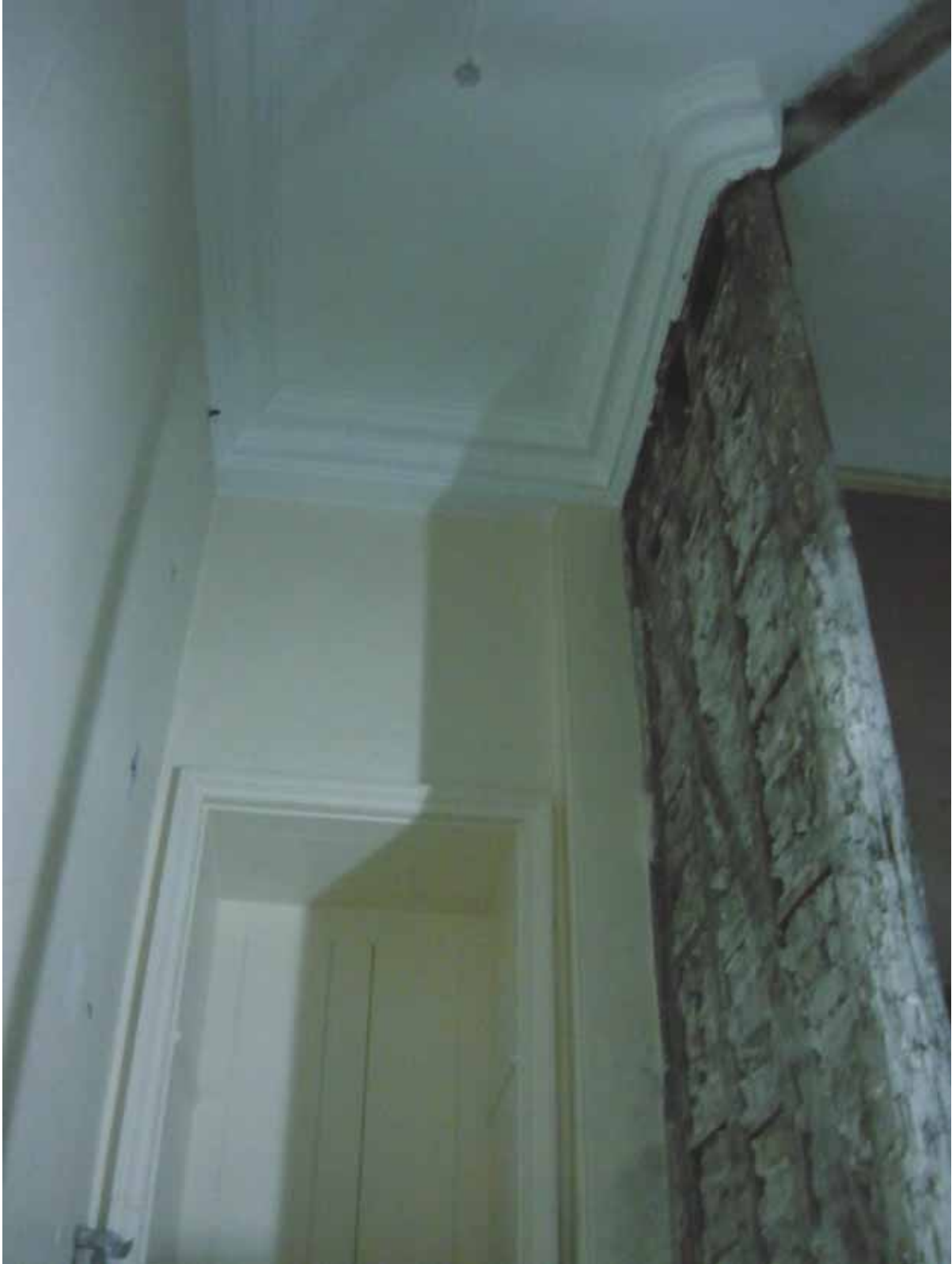
Plate 218: East end of the upper part of the south wall in Room M18 and upper part of the east wall of the rectangular (in plan) construction in the south-west corner of Room M18, looking south (EAF10 BHD6 (29))
