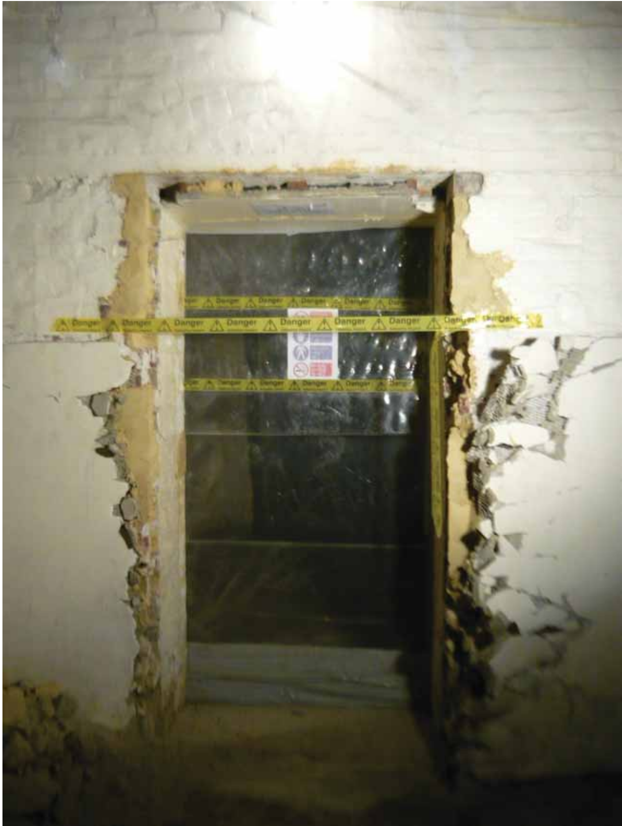
Plate 61: Doorway at the north end of the east wall in Room B48A, looking east (EAF10 BHD5 (5))
