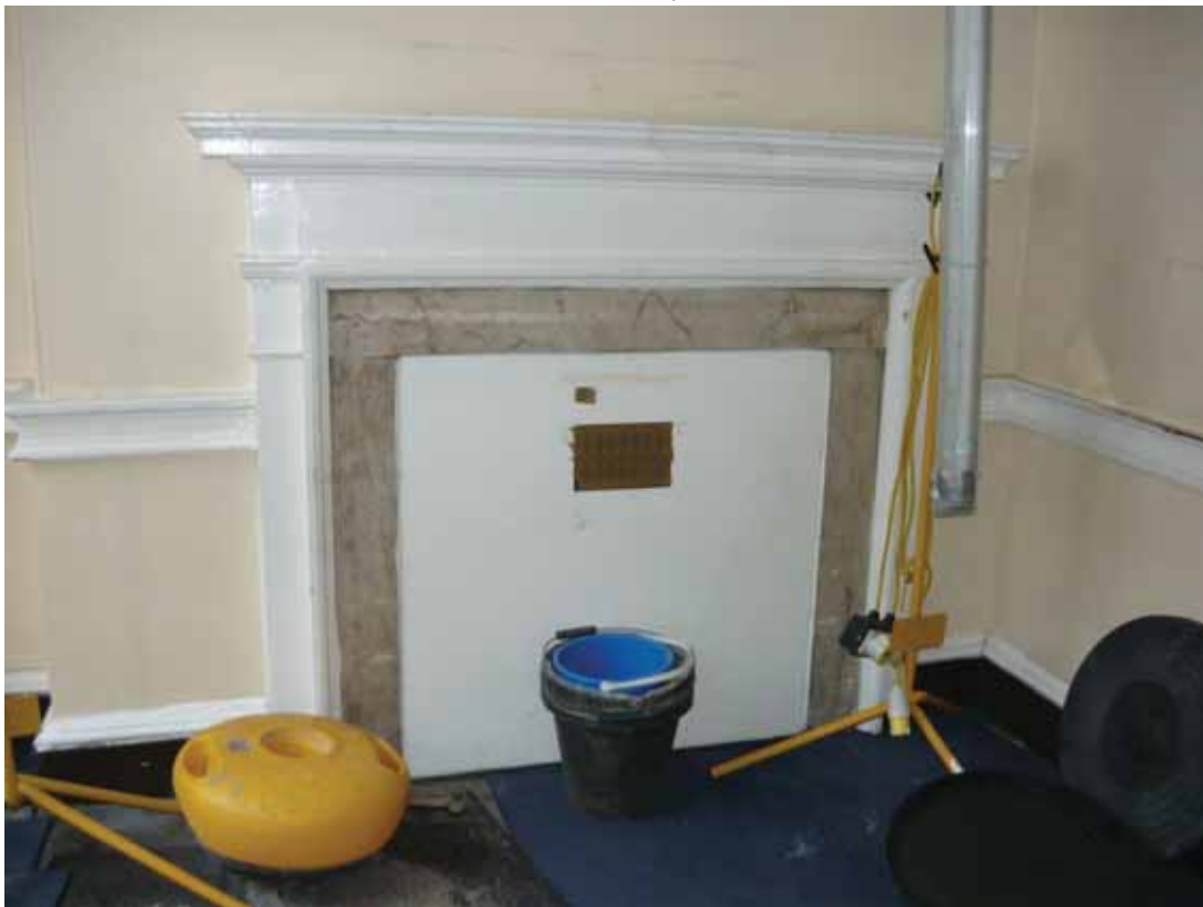
Plate 450: Fireplace (type 6) in the south wall of Room G28, looking south (EAF10 BHD1 (33))
