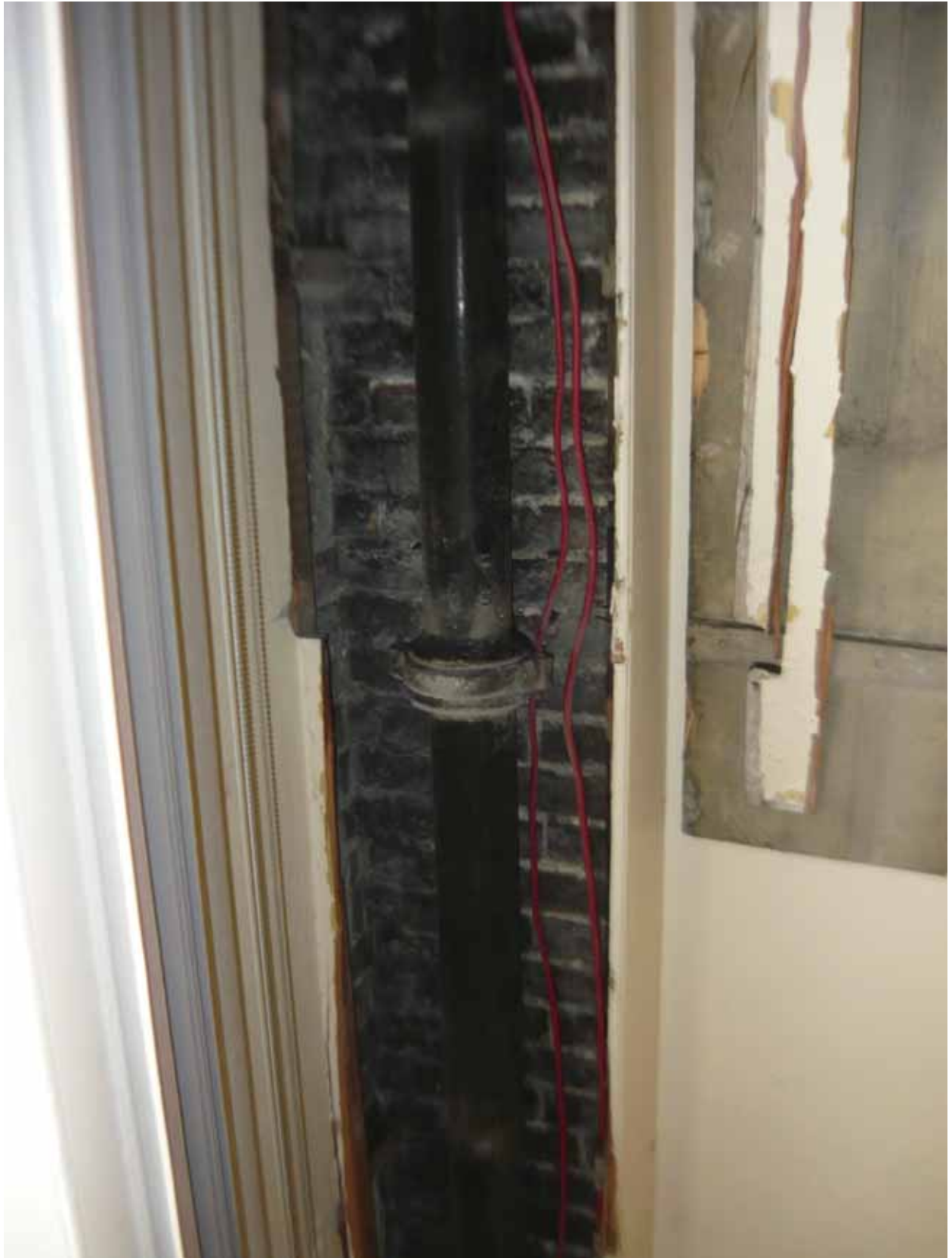
Plate 209: Cast iron pipe in the south-west corner of Room M15, looking south-west (EAF10 BHD2 (108))
