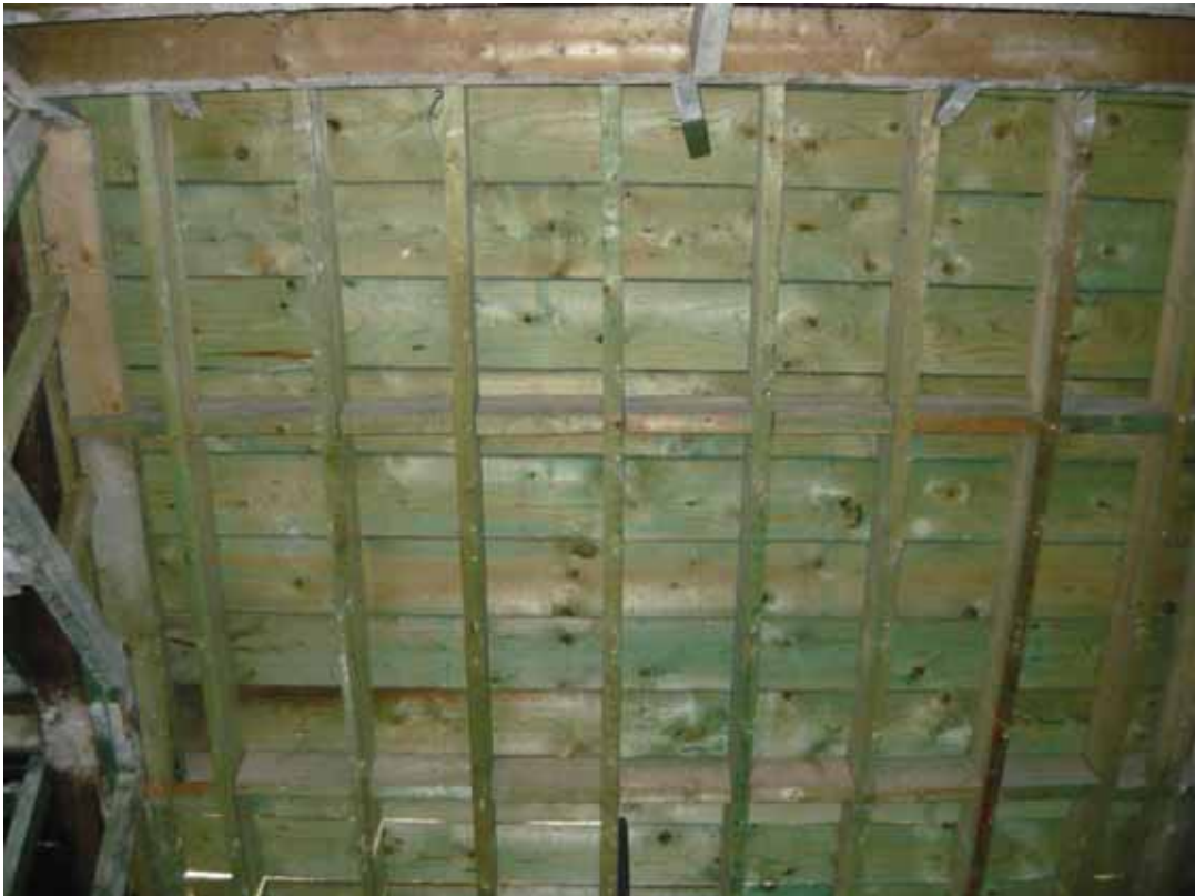
Plate 655: Replacement timbers in the roof above Room T120, looking east (EAF10 BHD10 (46))
