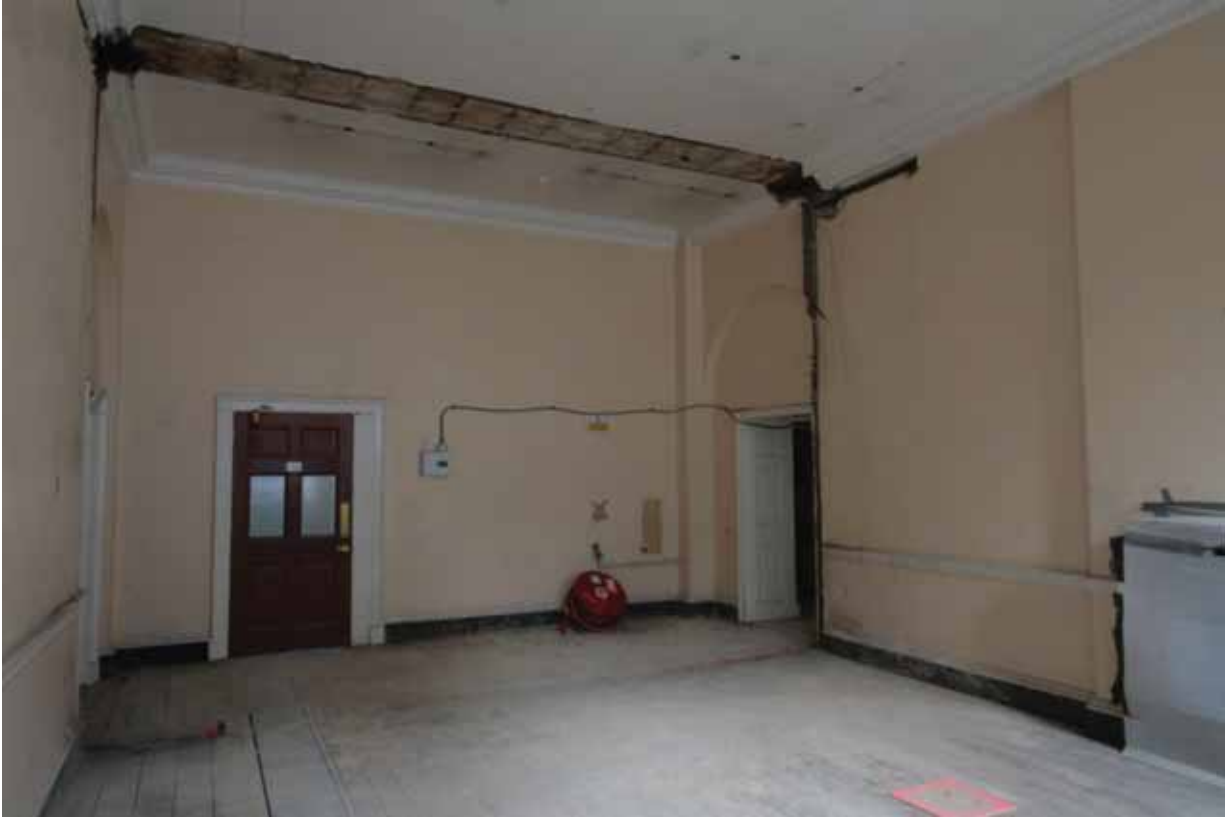
Plate 512: Removed partition wall between Corridor 09F and Room F63, looking north-west (EAF10 253)
