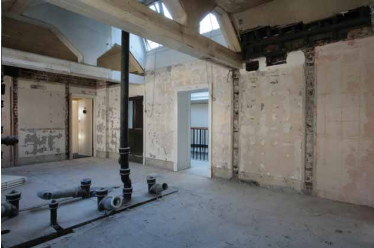
Plate 758: South (left) and west (right) walls in Room T20, looking south-west (EAF10 209)
