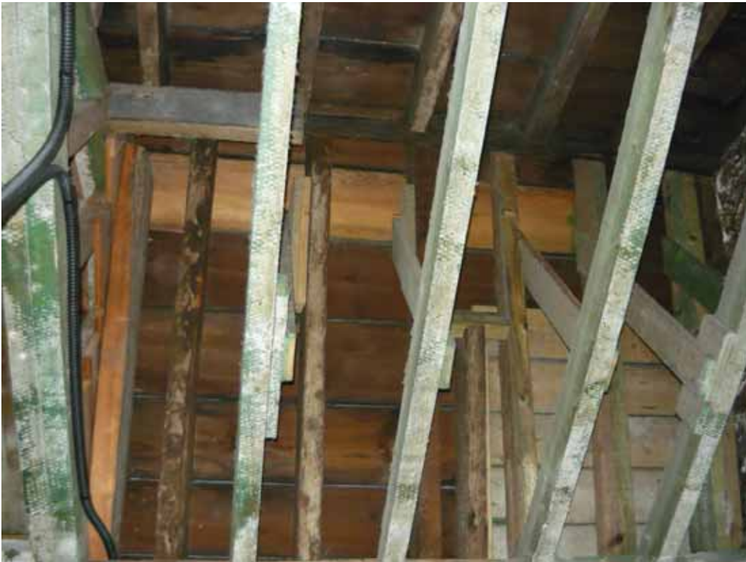
Plate 662: Roof structure at the south end of Room T119, looking east (EAF10 BHD10 (52))
