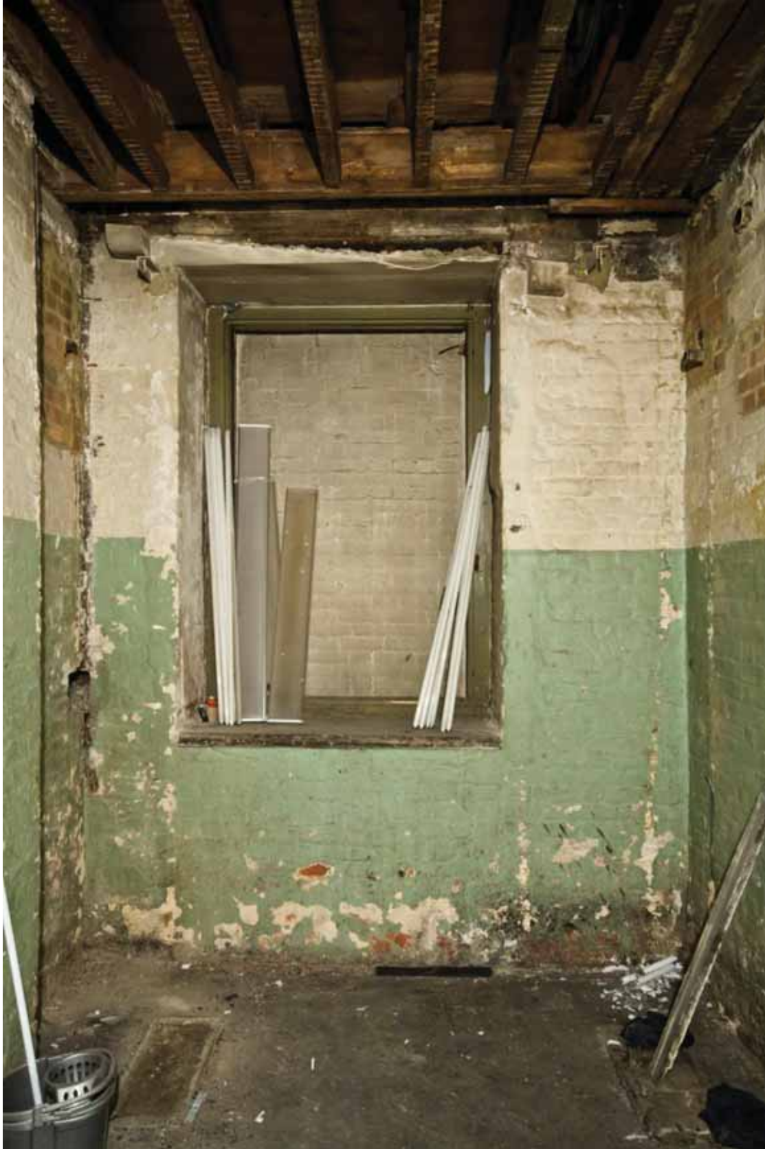
Plate 163: East wall of Room B54A, looking east (DSC_1491 _sitecode EAF10_© PCA Ltd 2010)
