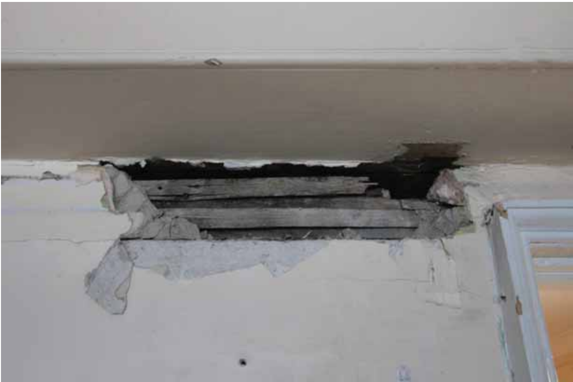
Plate 726: Area of removed plaster to the south of the doorway in the west partition wall in Room T115, looking west (EAF10 198)
