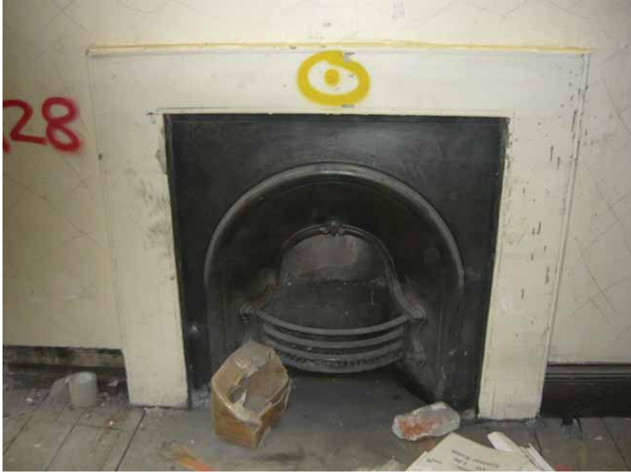
Plate 314: Fireplace in the south wall in Room M28, looking south (EAF10 BHD12 (23))
