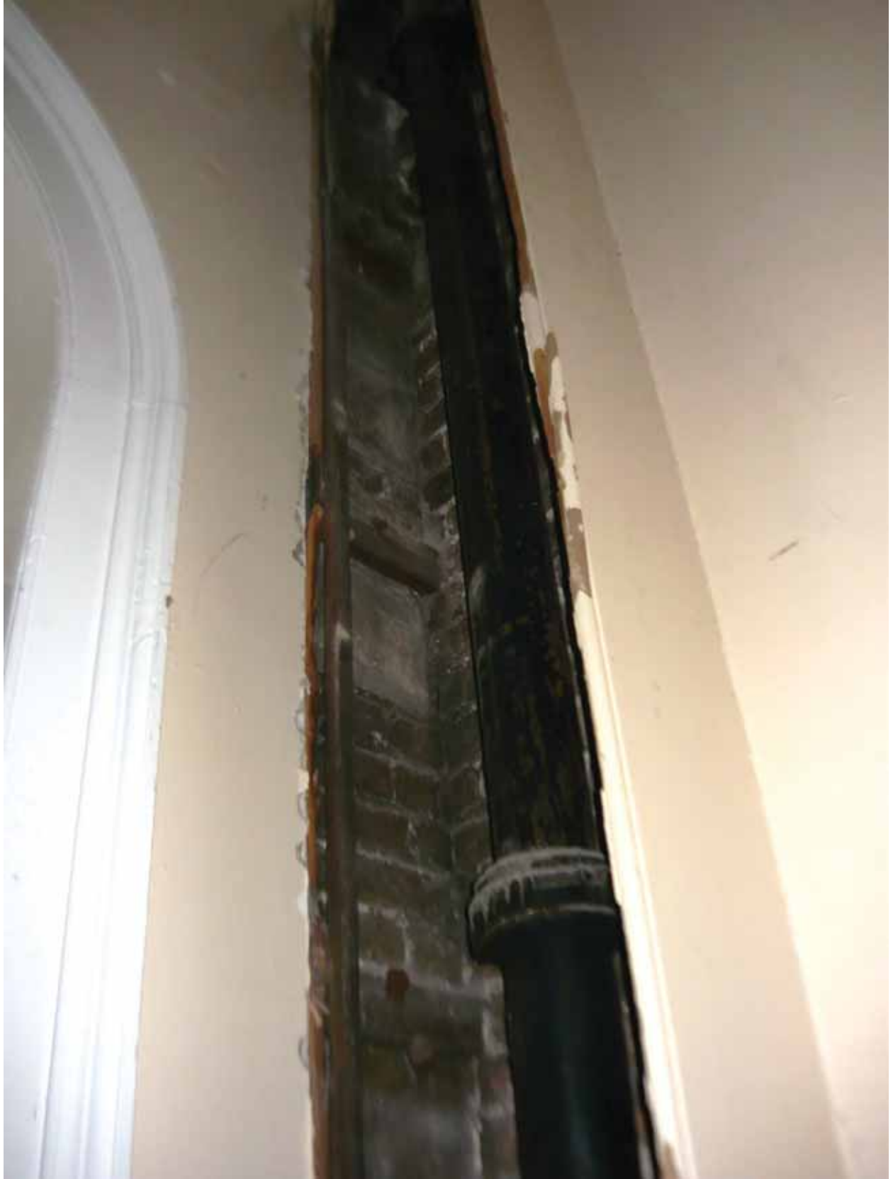
Plate 211: Cast iron pipe in the north-west corner of Room M16, looking north-west (EAF10 BHD3 (73))
