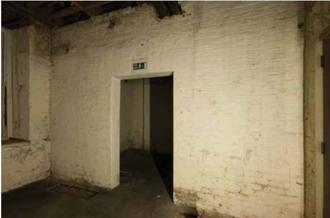
Plate 108: South wall of Room B49A, looking south-east (DSC_1403 _sitecode EAF10_© PCA Ltd 2010 _1)
