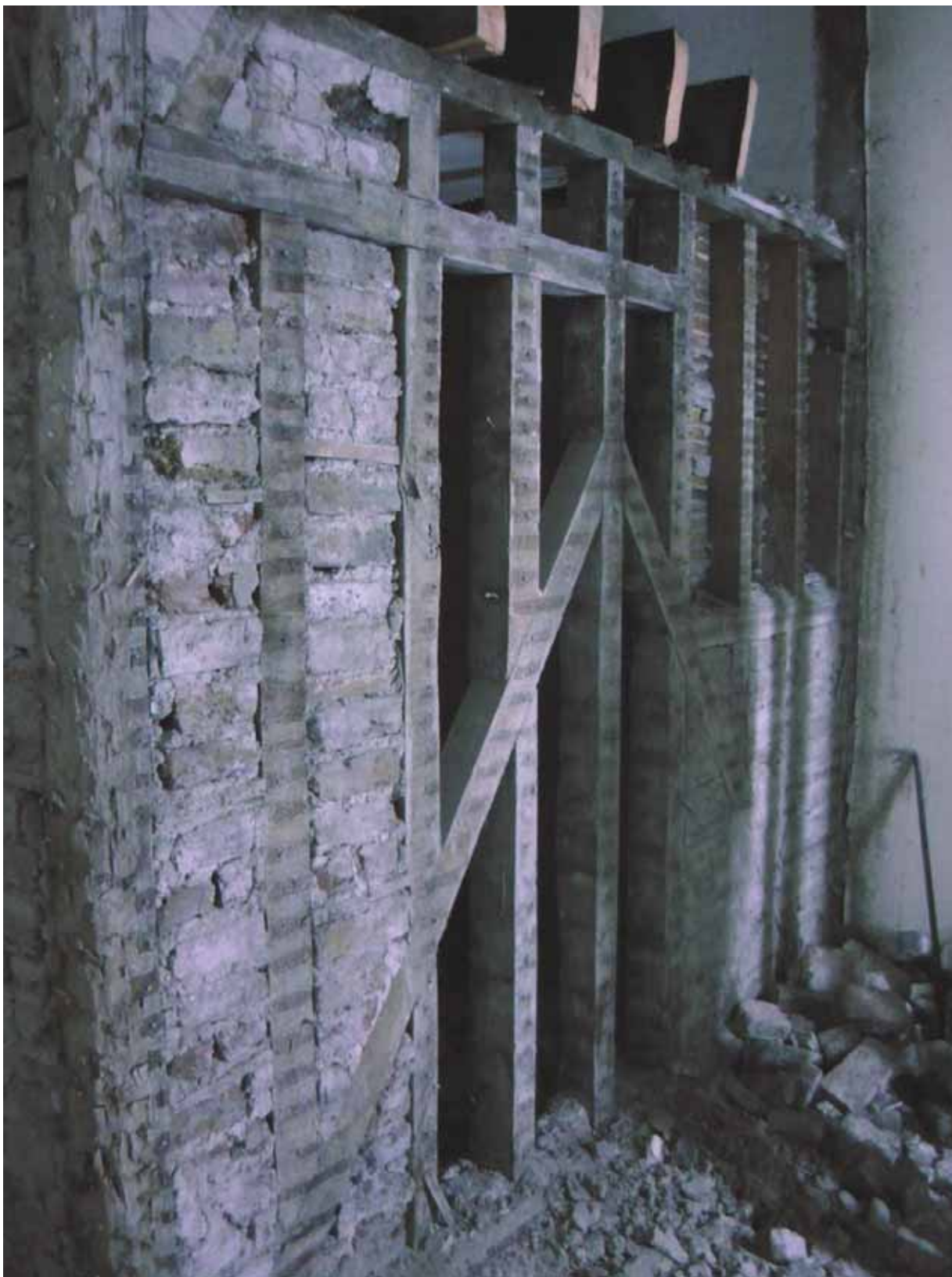
Plate 215: North wall of the rectangular (in plan) construction in south-west corner of Room M18, looking south-west (EAF10 BHD6 (26))
