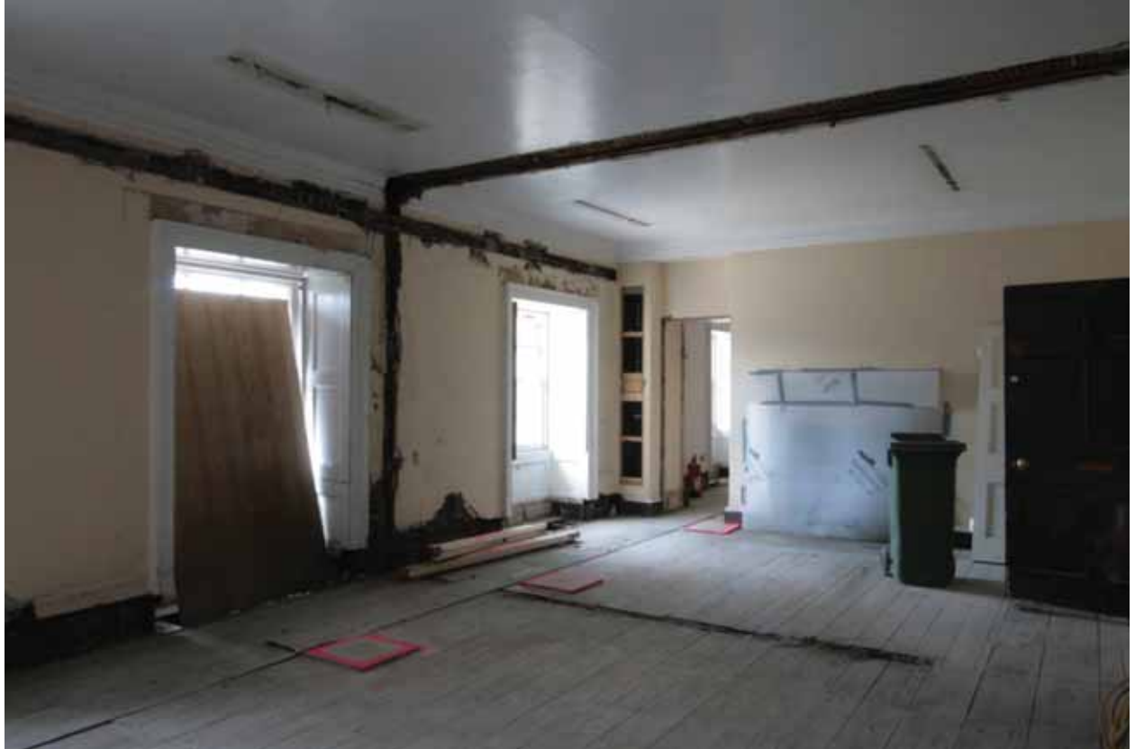
Plate 565: West (left) and north (right) walls in Room S02/S03, looking north-west (EAF10 230)
