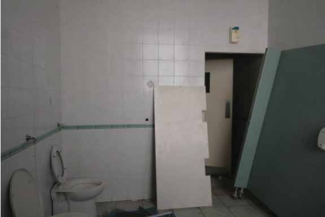
Plate 533: South partition (left), west partition (centre) and north (right) walls in Room F20, looking west (EAF10 185)
