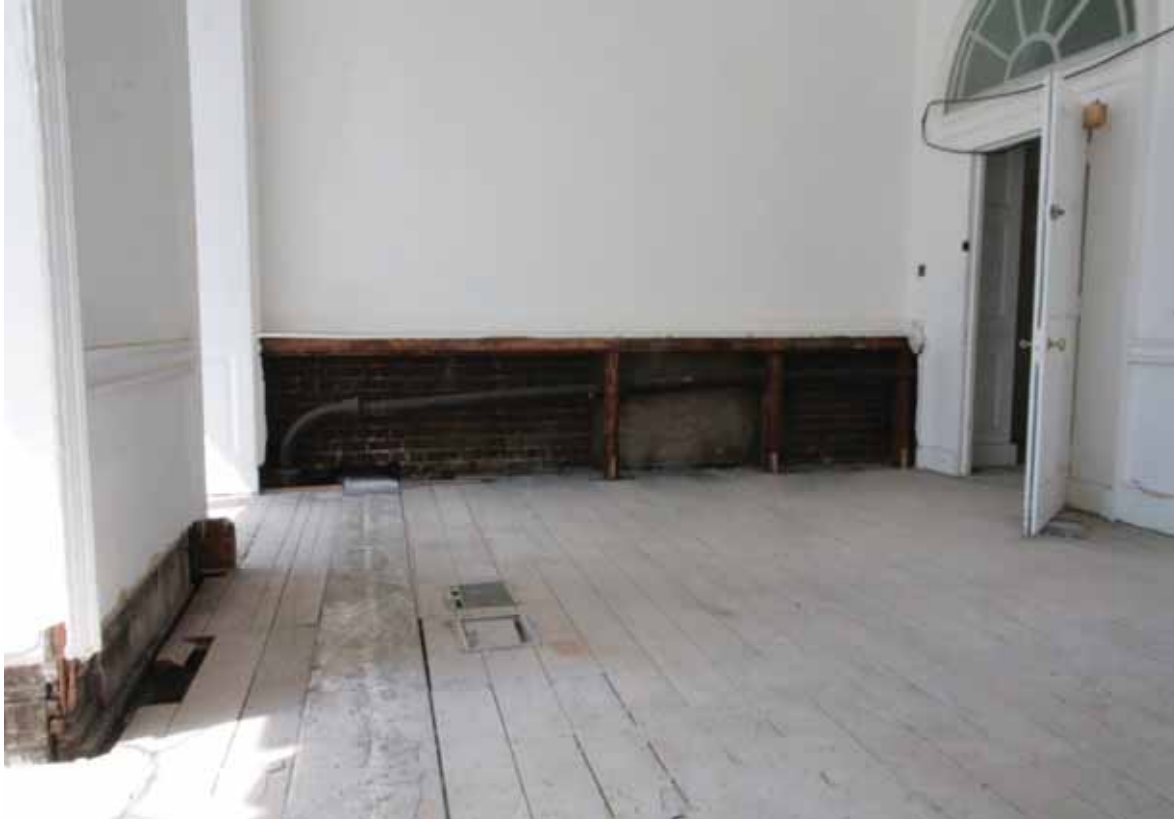
Plate 354: West (left), north (centre) and east (right) walls in Room G03, looking north (EAF10 272A)
