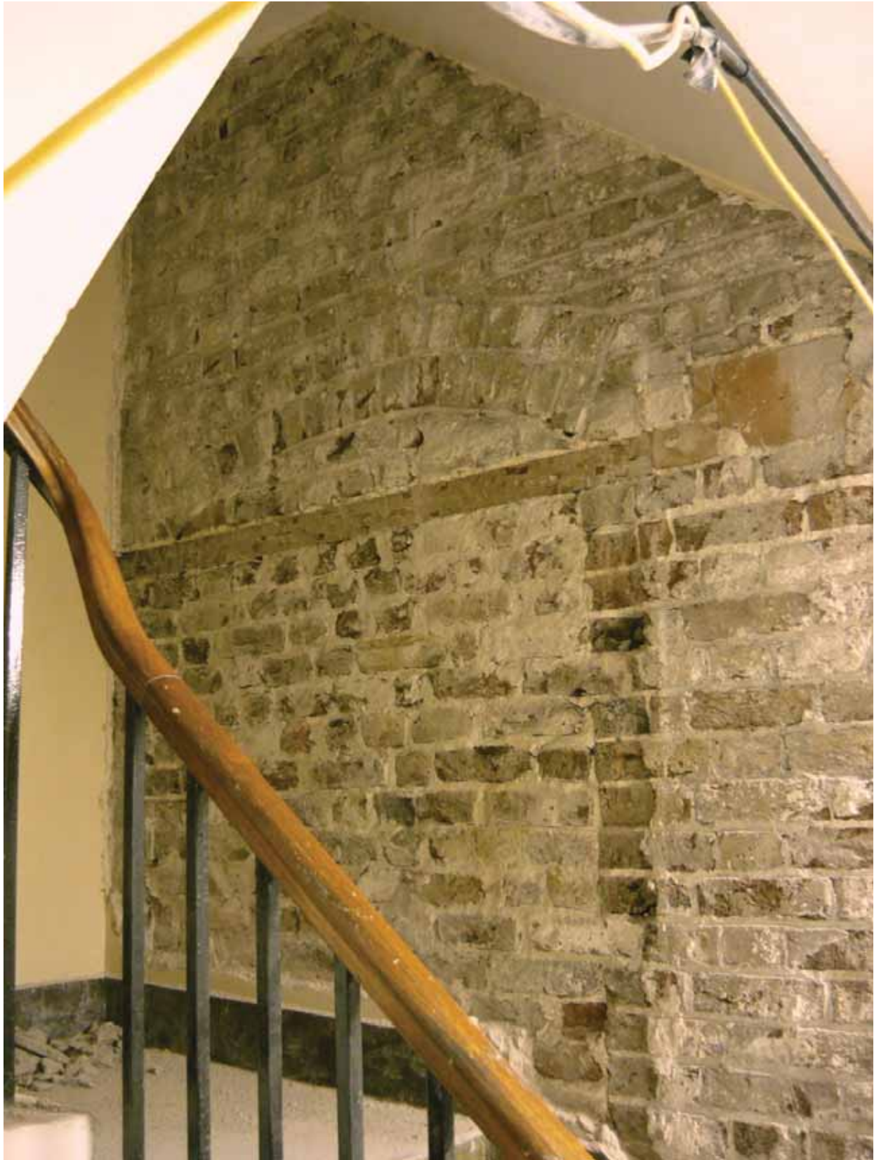
Plate 247: West (left) and north (centre and right) walls of Corridor 06LG looking north-west (EAF10 BHD6 (91))
