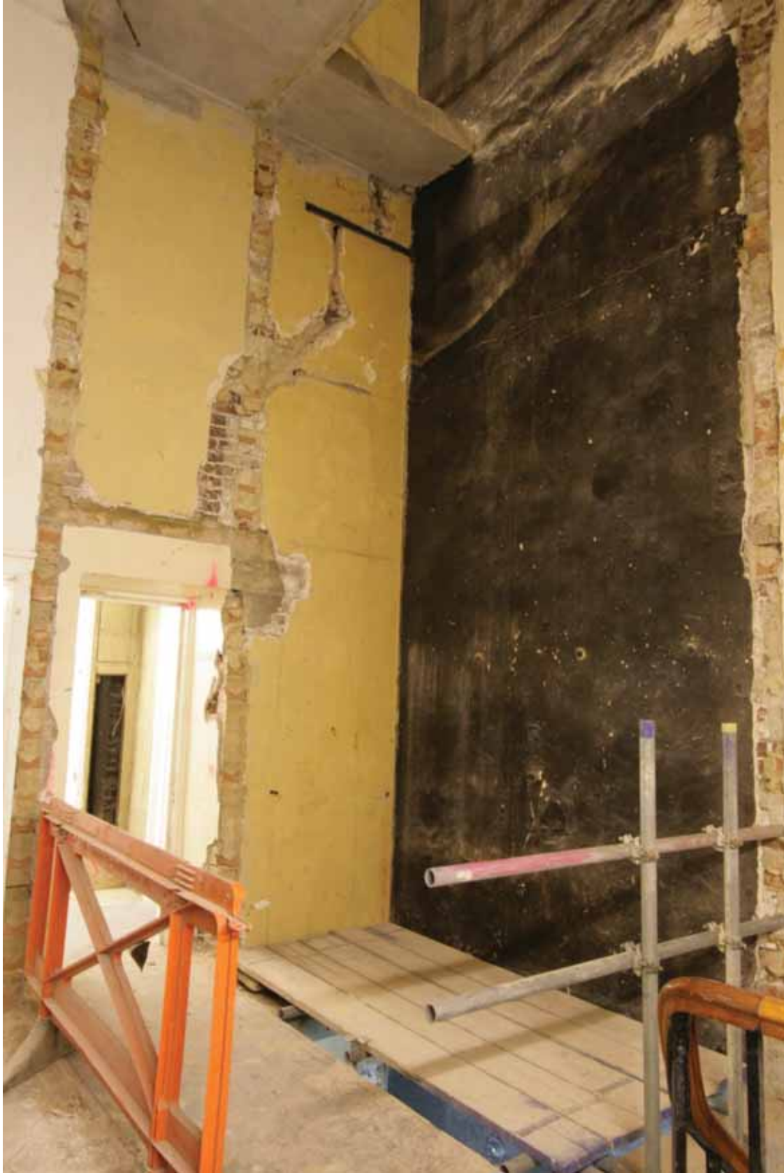
Plate 395: South (left) and west (right) walls of Corridor 08G, looking south-west (EAF10 A100 024)
