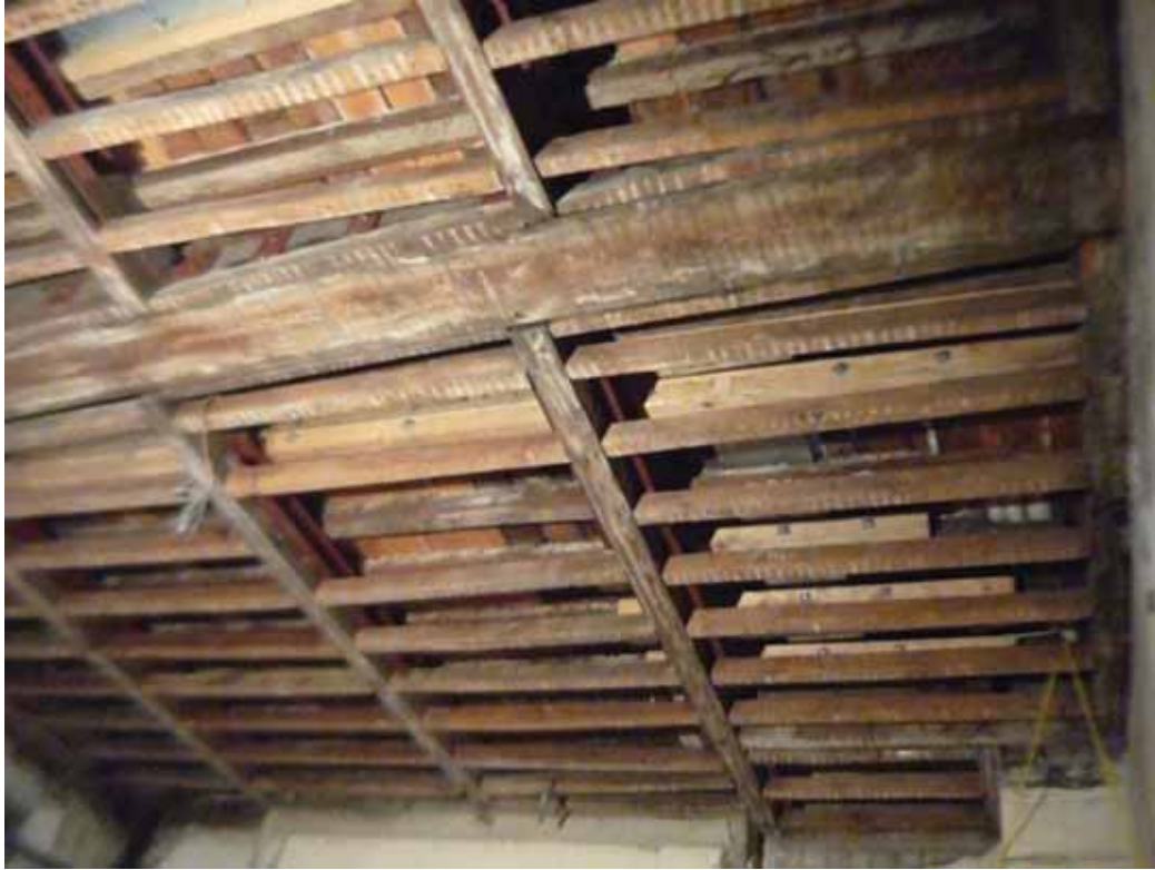
Plate 39: Primary and secondary floor joists visible following the removal of the lath and plaster ceiling in Room B47A, looking north (EAF10 BHD5 (86))
