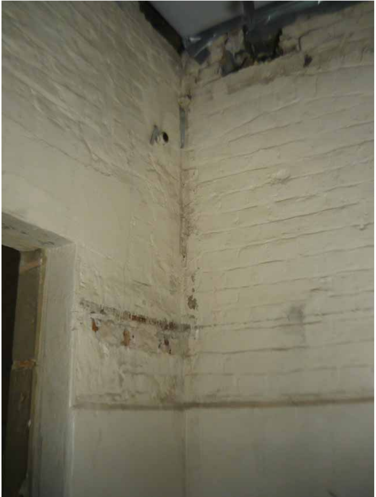
Plate 46: East (left) and south (right) walls of Room B48C, looking south-east (EAF10 BHD5 (40))
