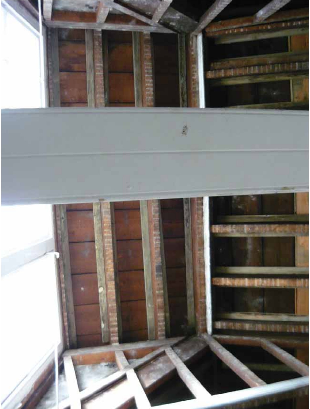
Plate 769: Dormer window in the west side of the roof above Room T23 (EAF10 BHD10 (18))
