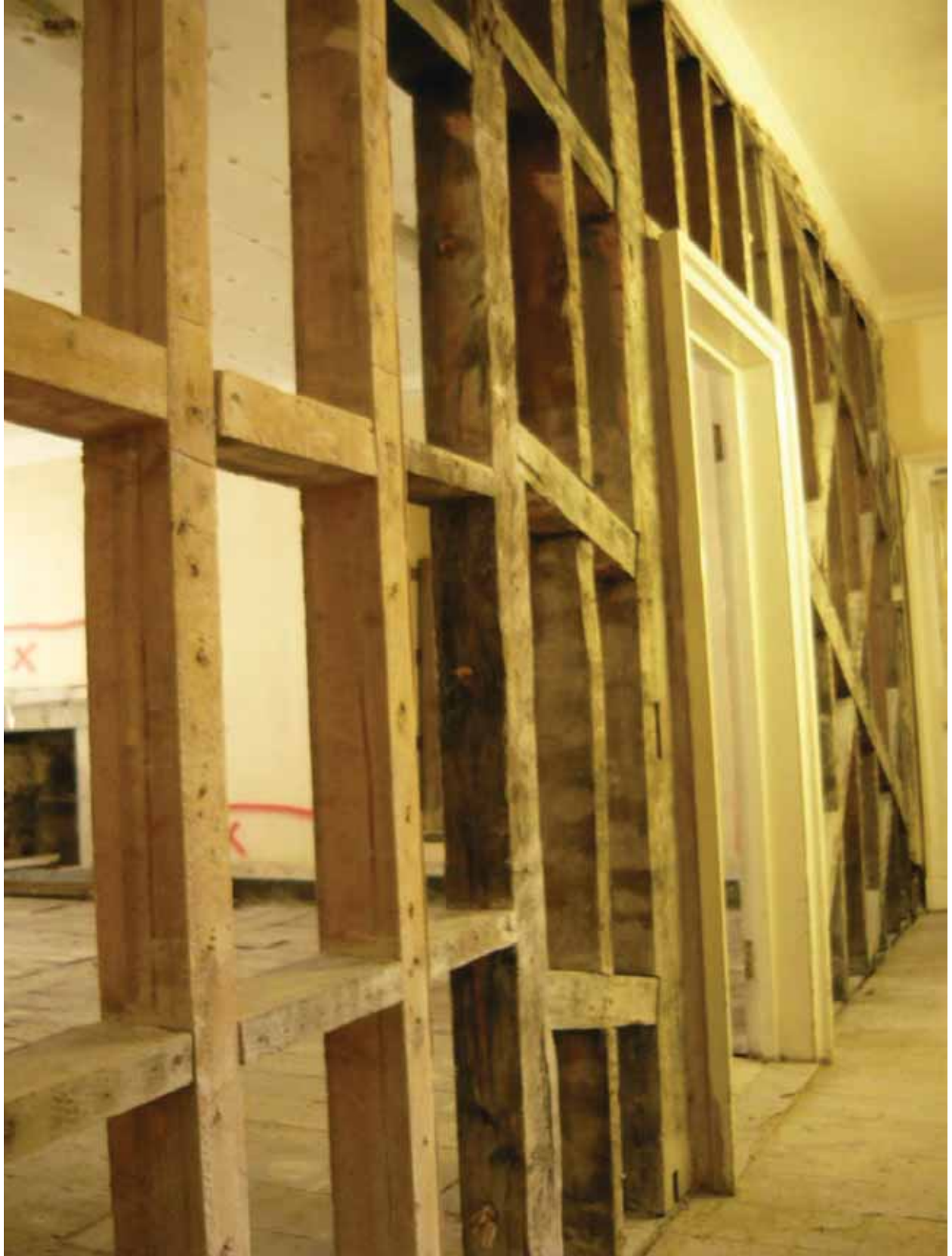
Plate 618: South (beyond) and east partition walls in Room S16, looking south-east (EAF10 BHD8 (37))
