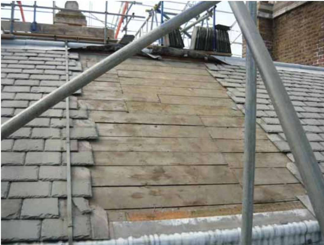
Plate 807: Slates stripped from the east side of the east roof over Room T16, looking east (EAF10 BHD9 (10))
