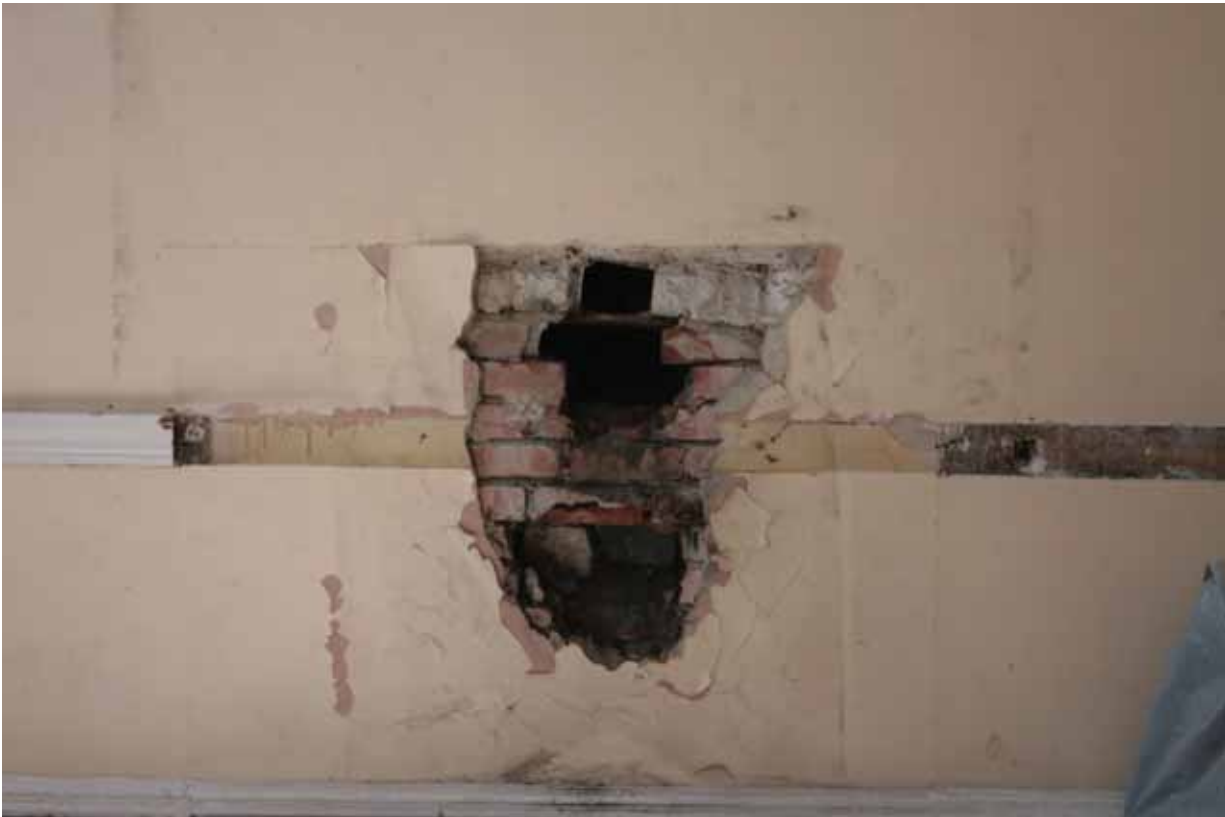
Plate 462: Infilled fireplace in the north wall of Room F01, looking north (EAF10 245)
