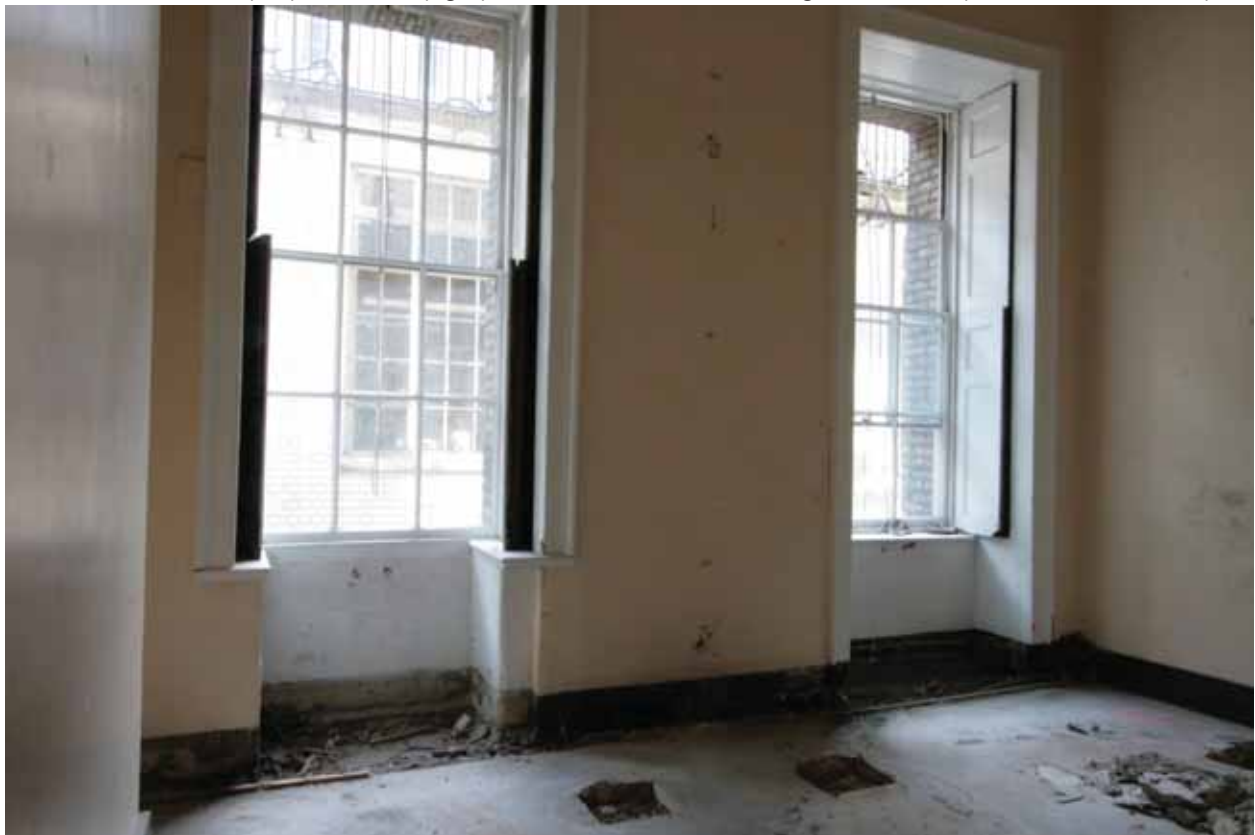
Plate 268: Windows in the east wall of Room M20, looking east (EAF10 287a)
