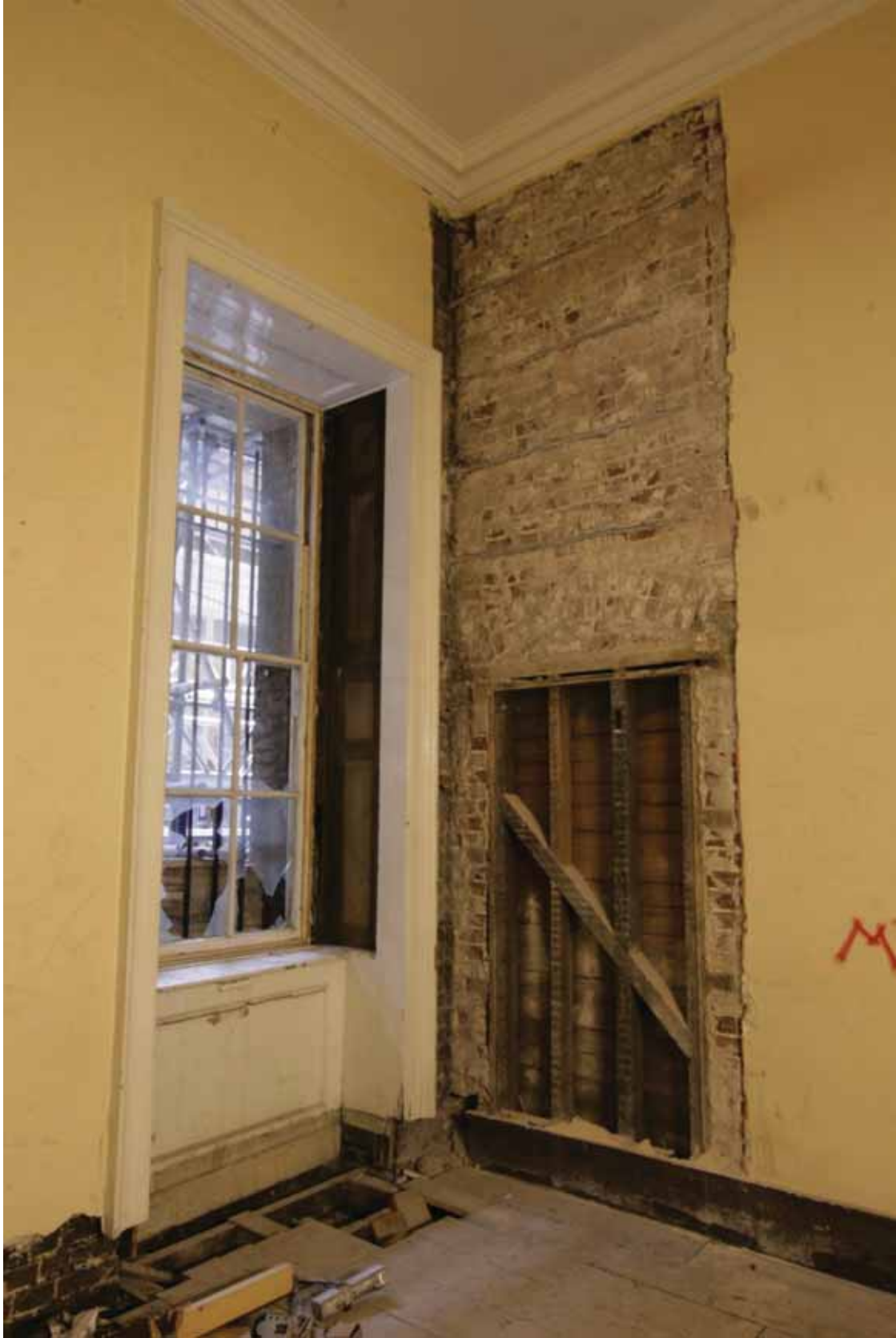
Plate 294: East (left) and south (right) walls in Room M25, looking south-east (EAF10 A100 031)
