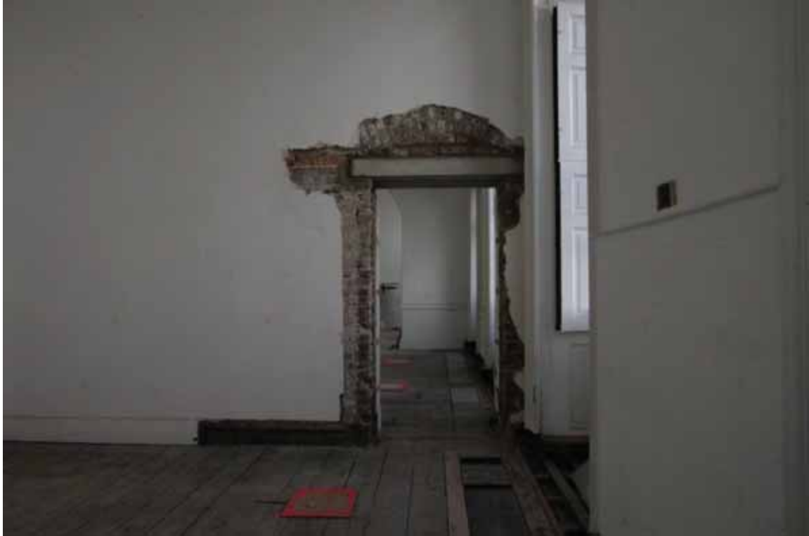
Plate 406: Doorway opened up at the east end of the north wall of Room G40, looking north (EAF10 278)
