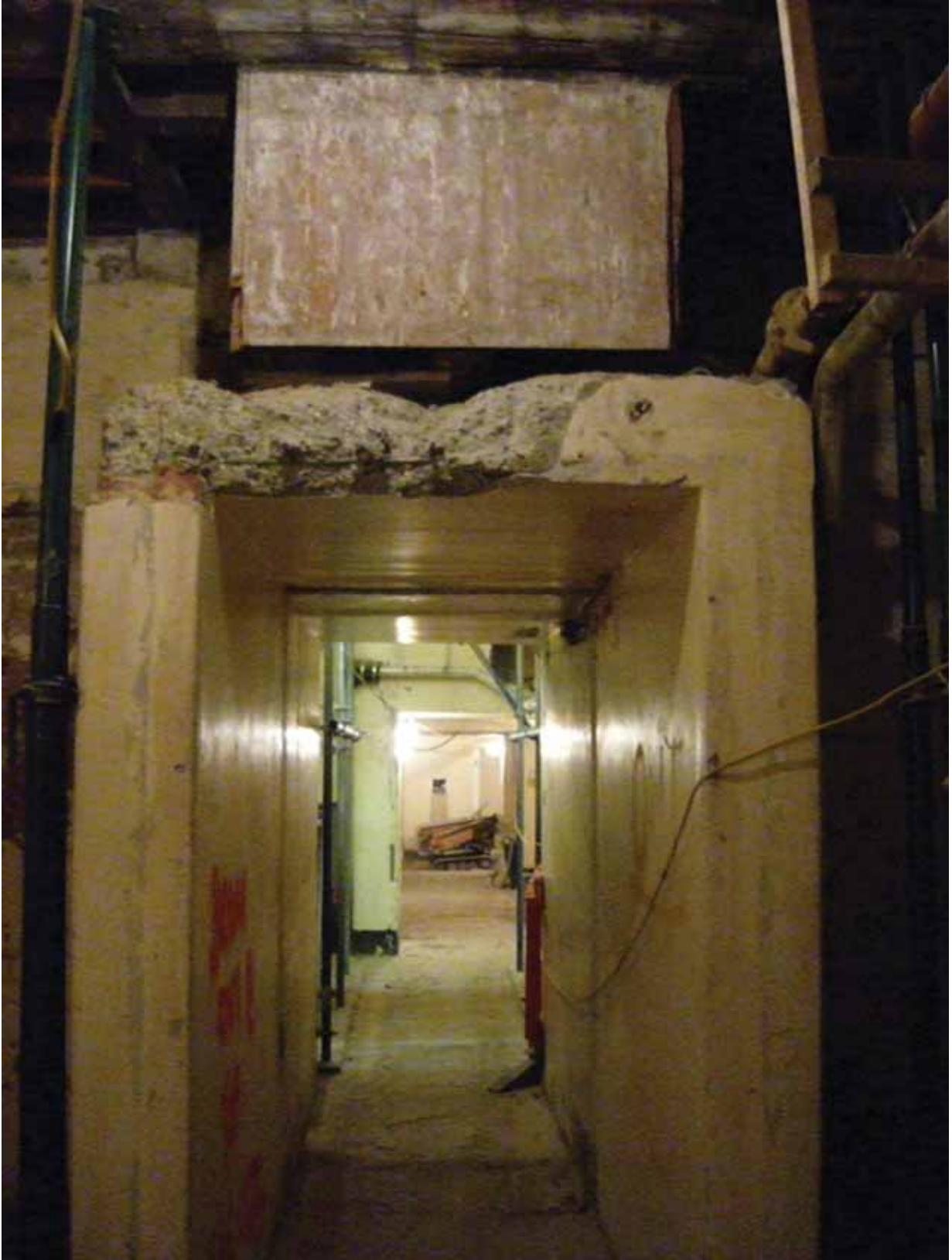
Plate 68: South doorway in Room B63 during the removal of its concrete surround, looking south (EAF10 BHD6(1))
