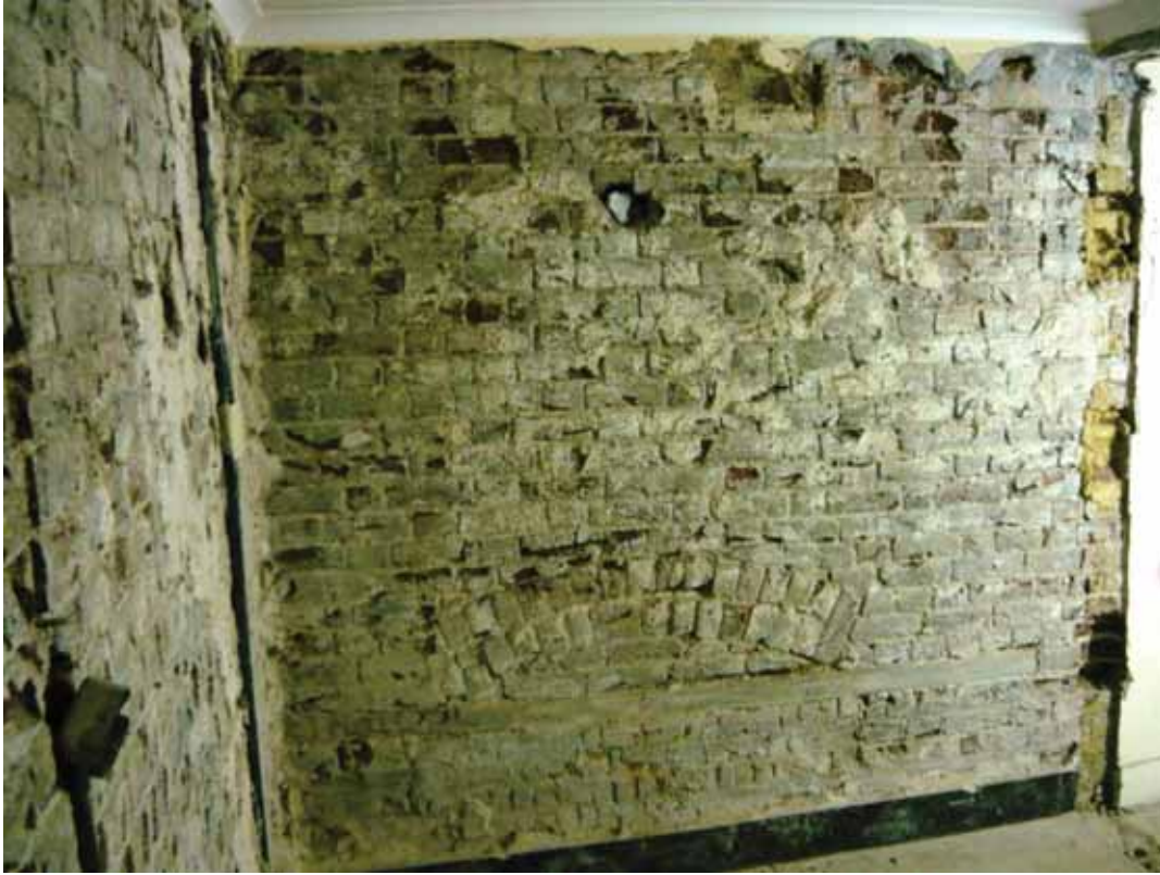
Plate 249: North end of the east wall (upper level) in Corridor 06LG looking east (EAF10 BHD7 (10))
