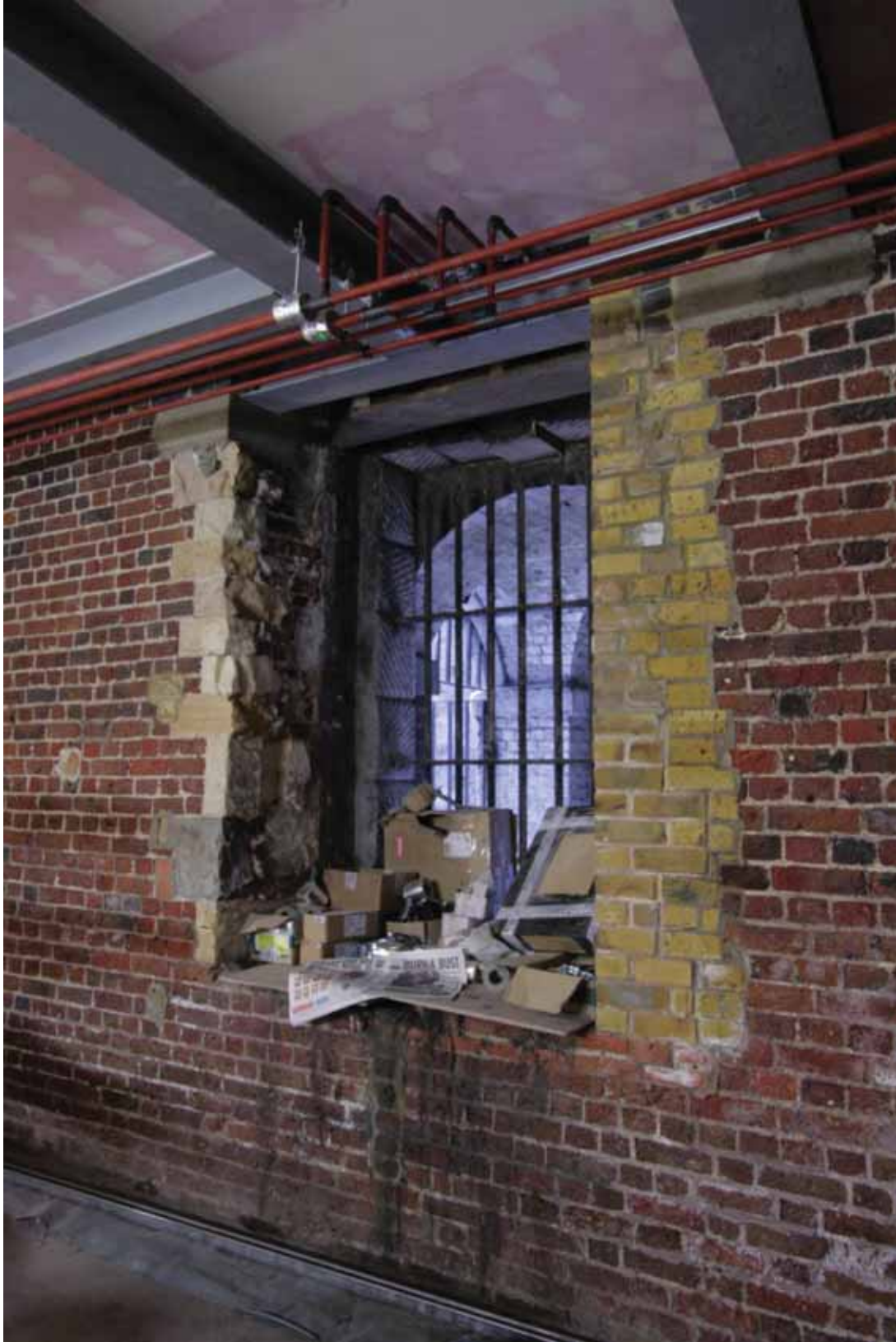
Plate 53b: Window opening reinstated during the current work in the west wall of Room B48A and B48C, looking south-west (N.B. the yellow brick is 2011 work) (EAF10 A-D101 003)
