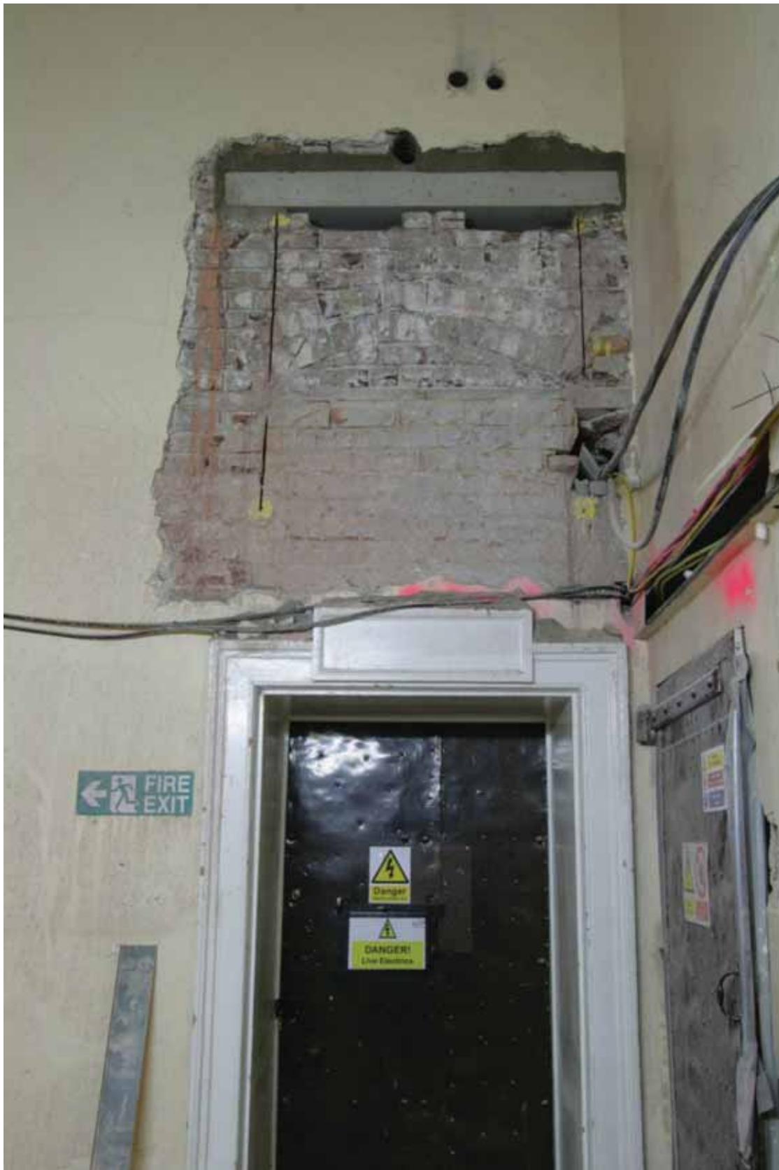
Plate 233: Doorway at the north end of the west wall of Corridor 04LG, looking west (EAF10 A100 029)
