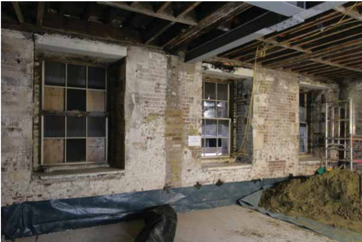
Plate 33: West wall of Rooms B47A and B47C following removal of the dividing wall, looking north-west (EAF10 A100 034)
