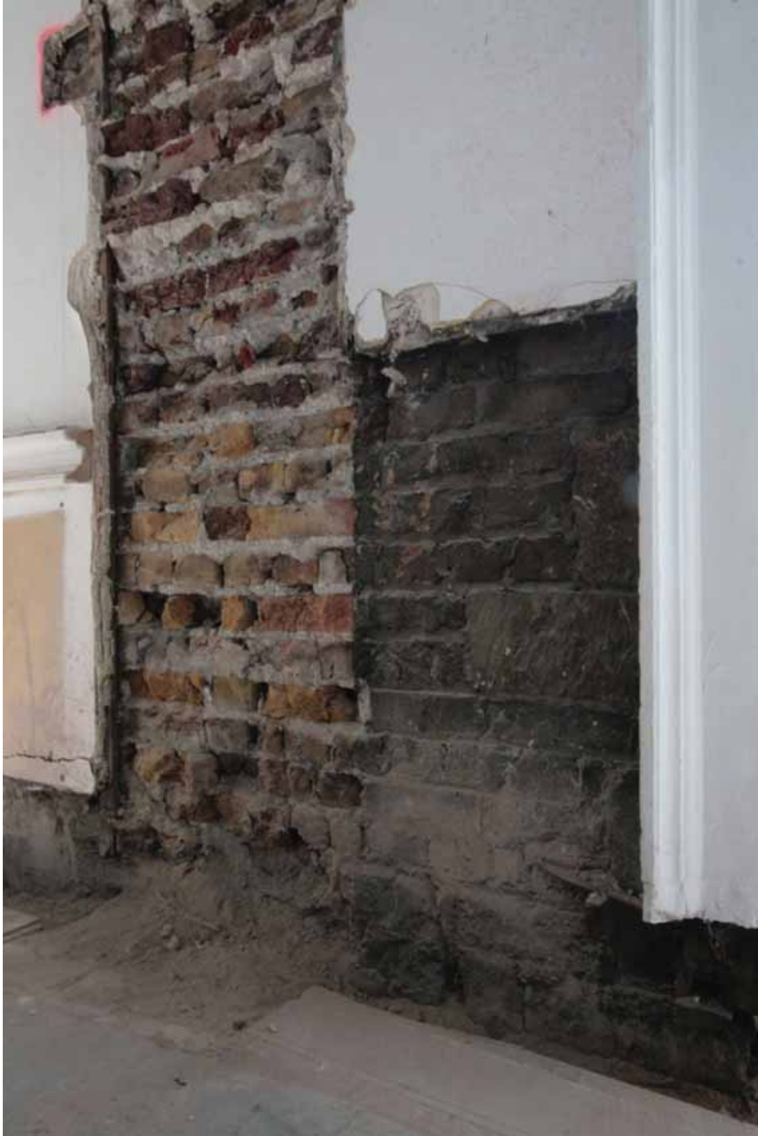
Plate 366: South-west corner of Room G06 with west end of south wall removed (left) and wall covering removed from south end of west wall (right), looking south-west (EAF10 270)
