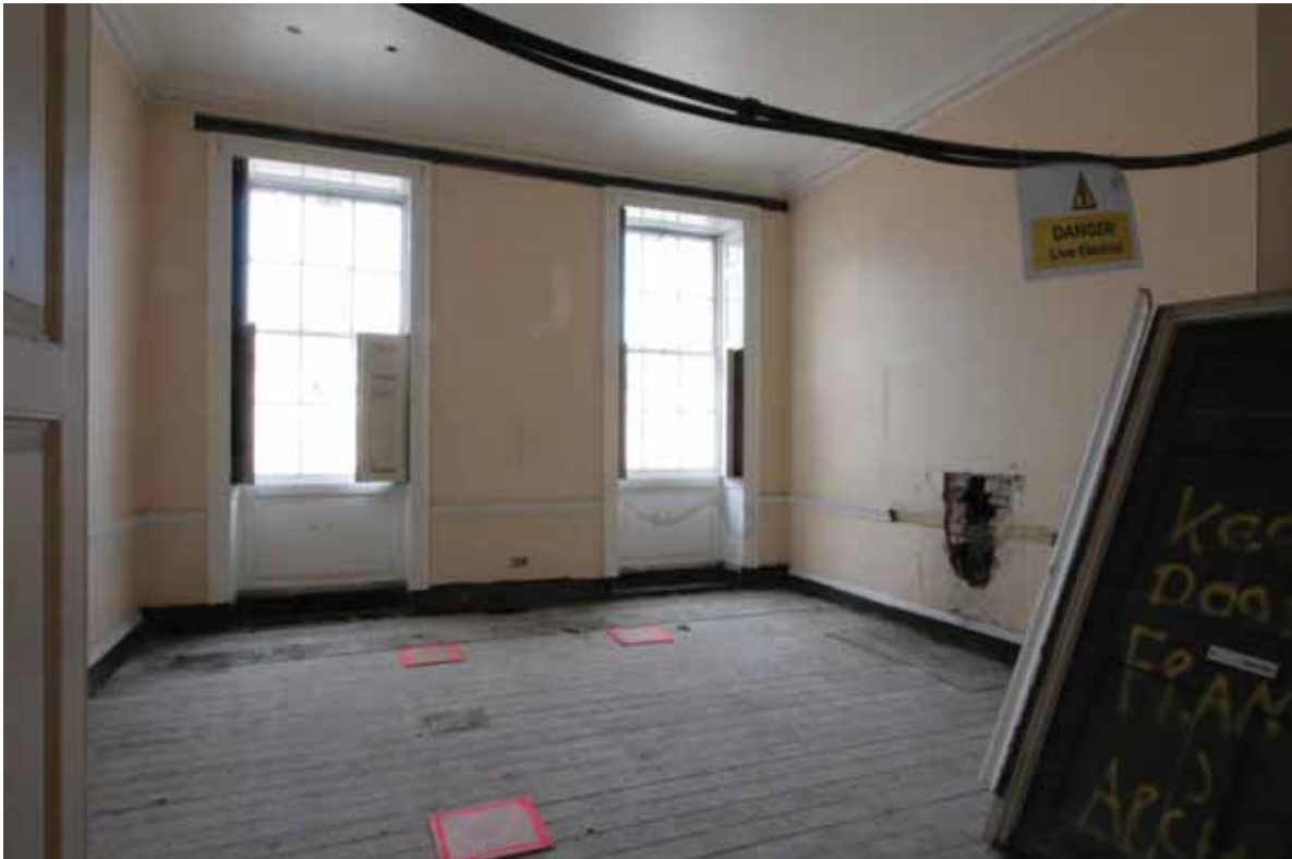
Plate 460: South (far left), west (centre) and north (right) walls in Room F01, looking west (EAF10 247A)
