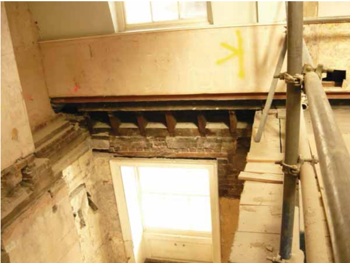
Plate 762: North (left) and east (right) walls in Room T20, looking north-east (EAF10 BHD8 (95))
