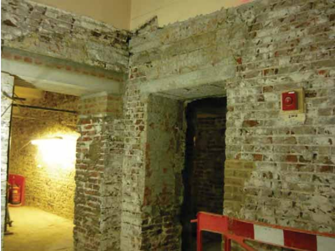
Plate 107a: North (left) and east (right) walls of Corridor 7, looking north-east; note north doorway lintel and inserted brickwork is 2011 work (EAF10 BHD13 (17))
