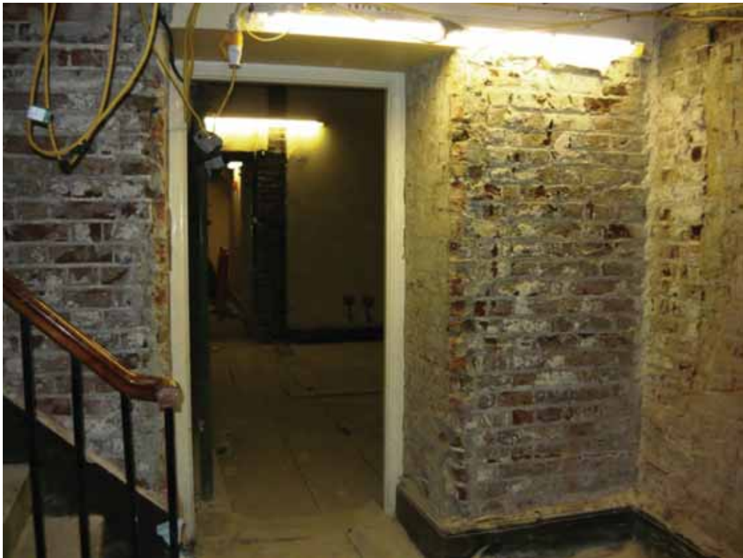
Plate 254: North (left and centre) and east (right) walls of Corridor 06LG looking north (EAF10 BHD7 (17))
