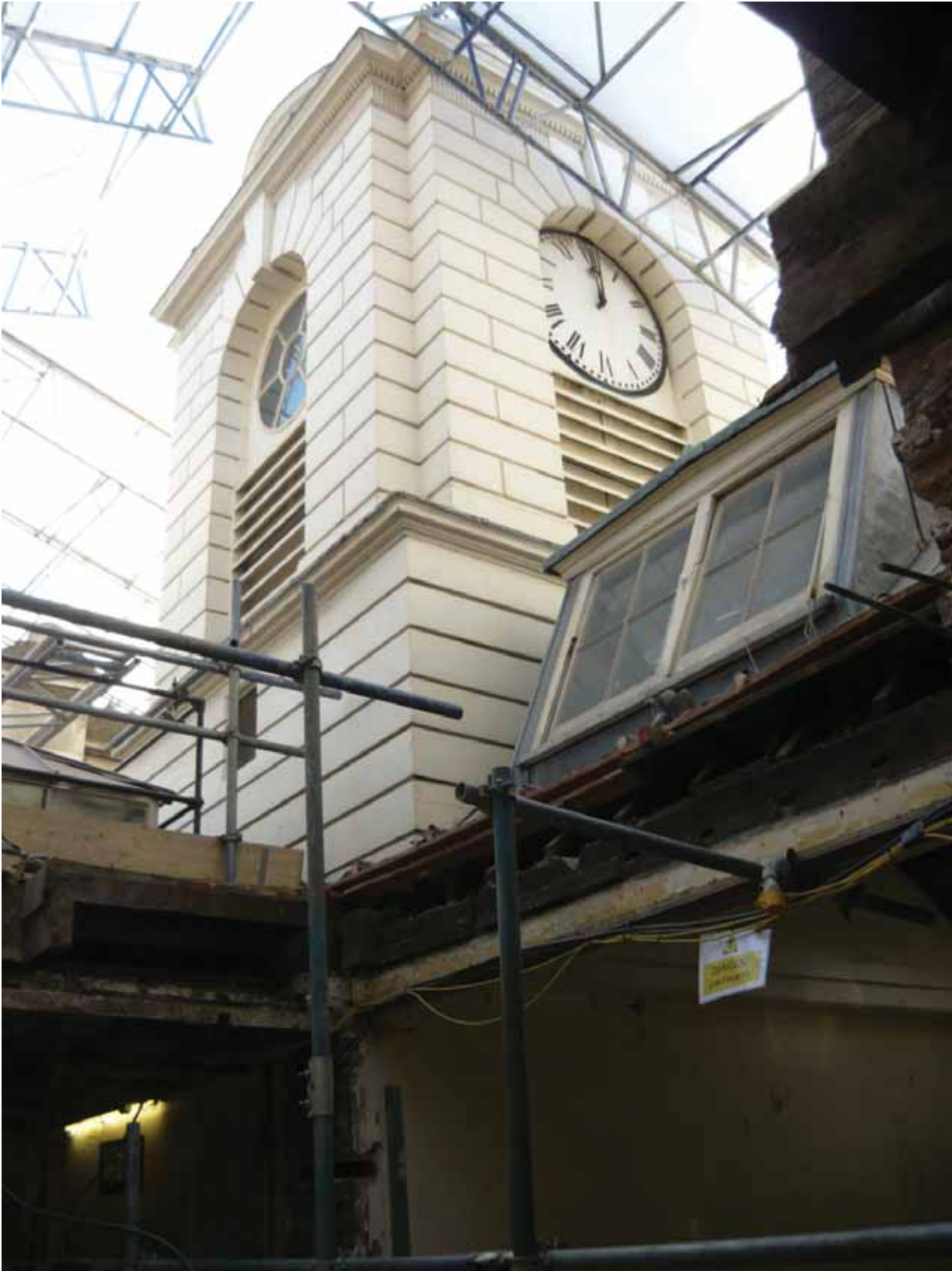
Plate 802: Clock tower over Room T04 and dormer window over Room T05, looking south-west (EAF10 BHD8 (54))
