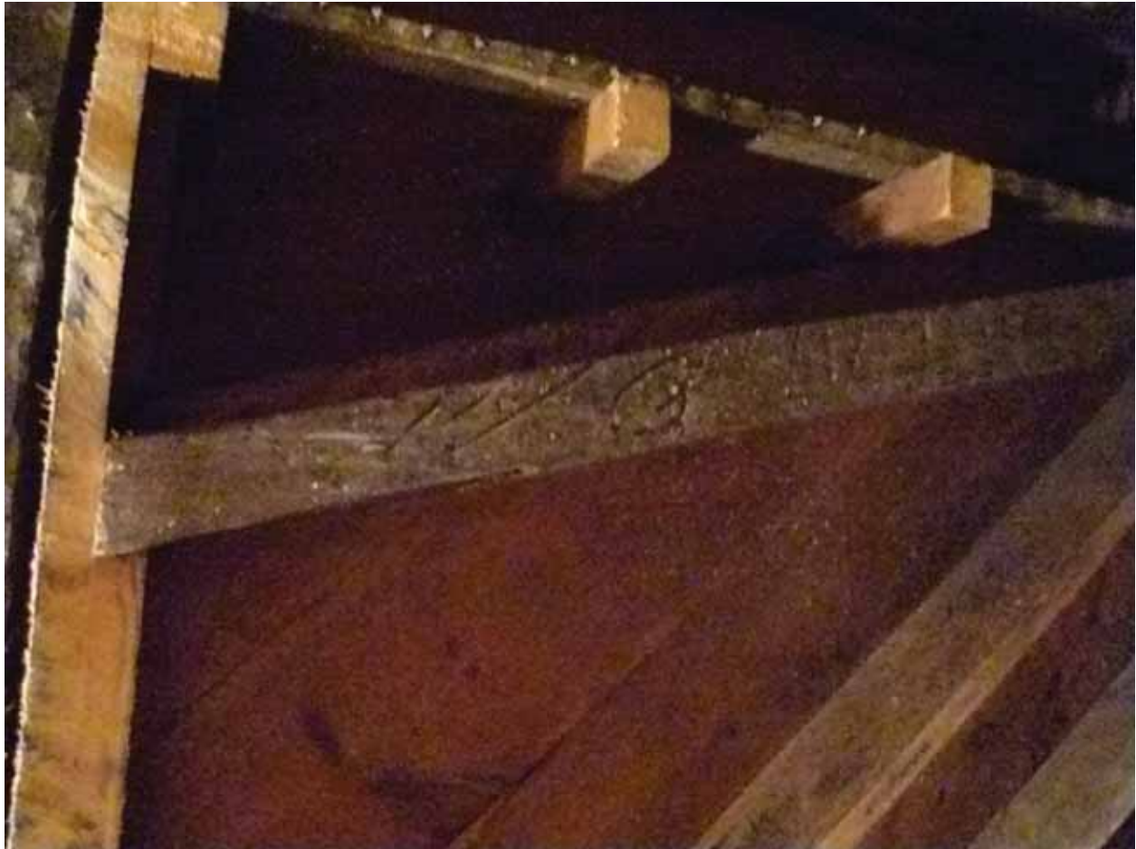
Plate 71: Inscribed marks on the soffit of one of the timbers of the inserted staircase above the concrete surround to the south doorway in Room B63, looking up and south (EAF10 BHD6(12))
