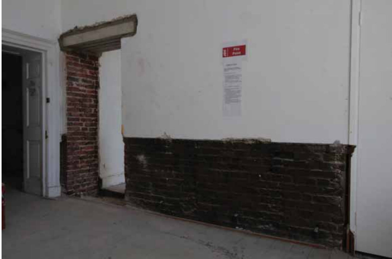
Plate 376: East (left) and south (right) walls in Room G09, looking south-east (EAF10 265)
