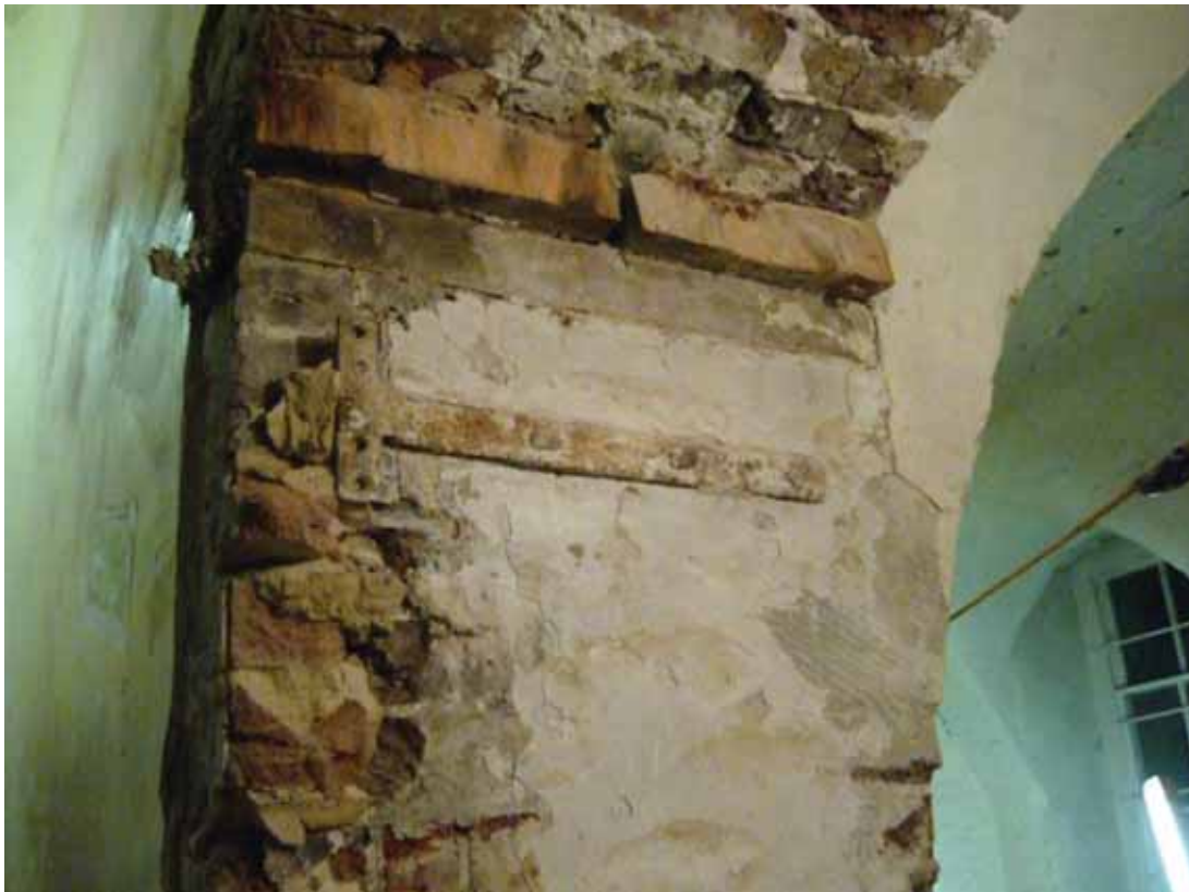
Plate 76: North side of east doorway in Stairs 01, looking north-east into Room B50 (EAF10 BDH6(68))
