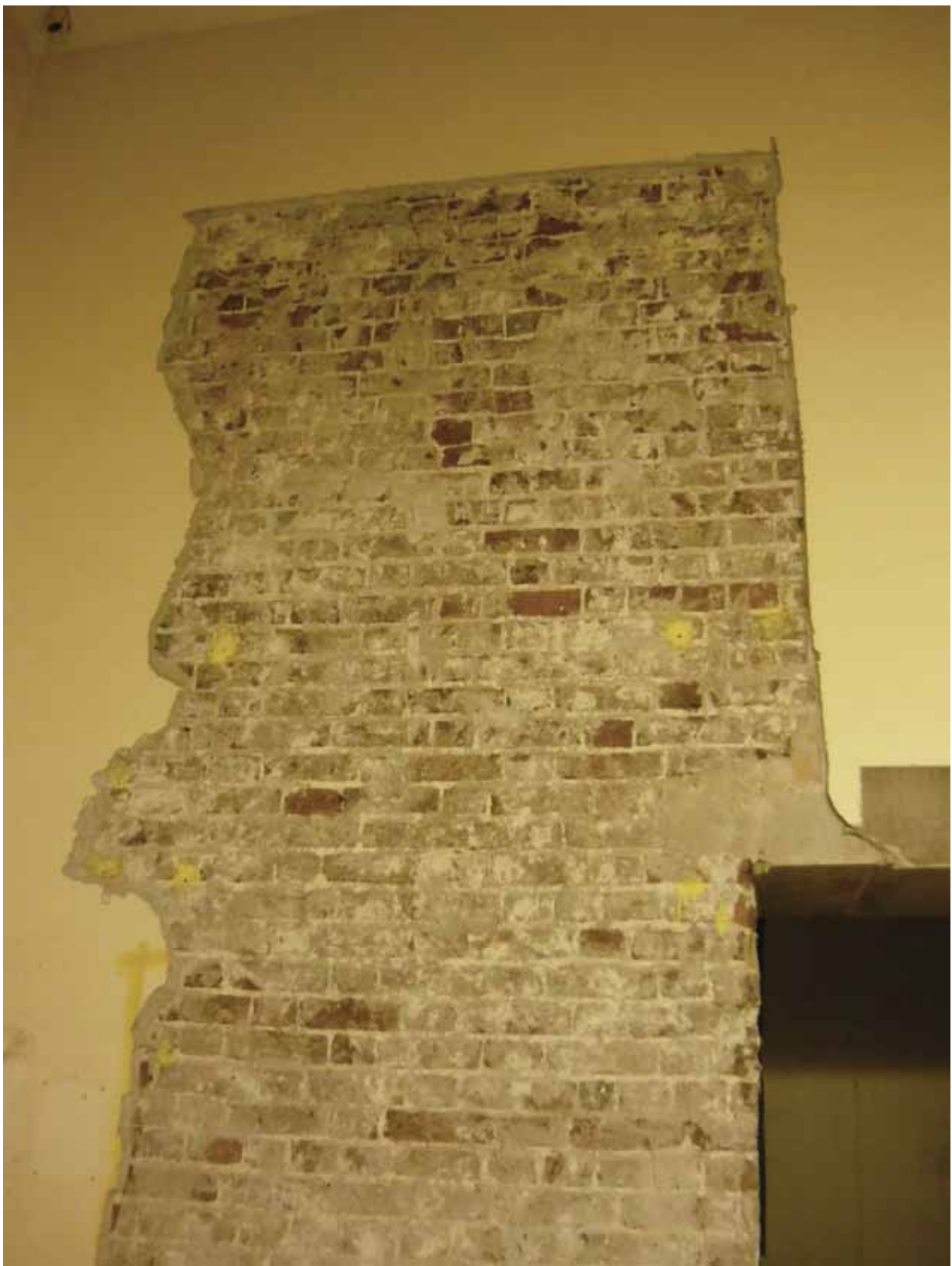
Plate 239c: Stripping of plaster from the south side of the west doorway in Corridor 05LG looking west (EAF10 BHD6 (20))
