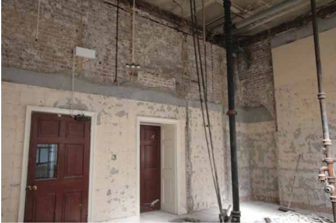
Plate 424: West (left) and north (right) walls in Room G20, looking north-west (EAF10 283a)
