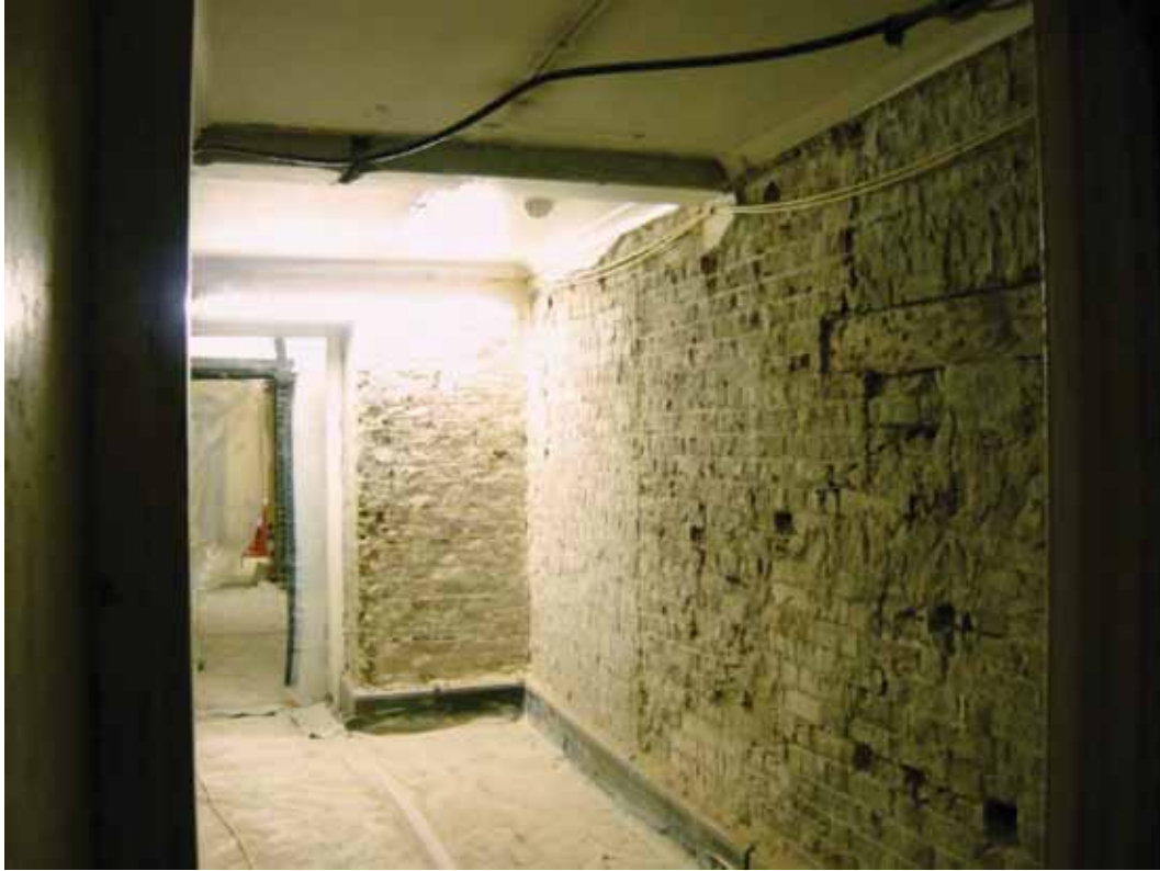
Plate 243: North (left) and east (right) walls of Corridor 06LG looking north-east (EAF10 BHD6 (87))
