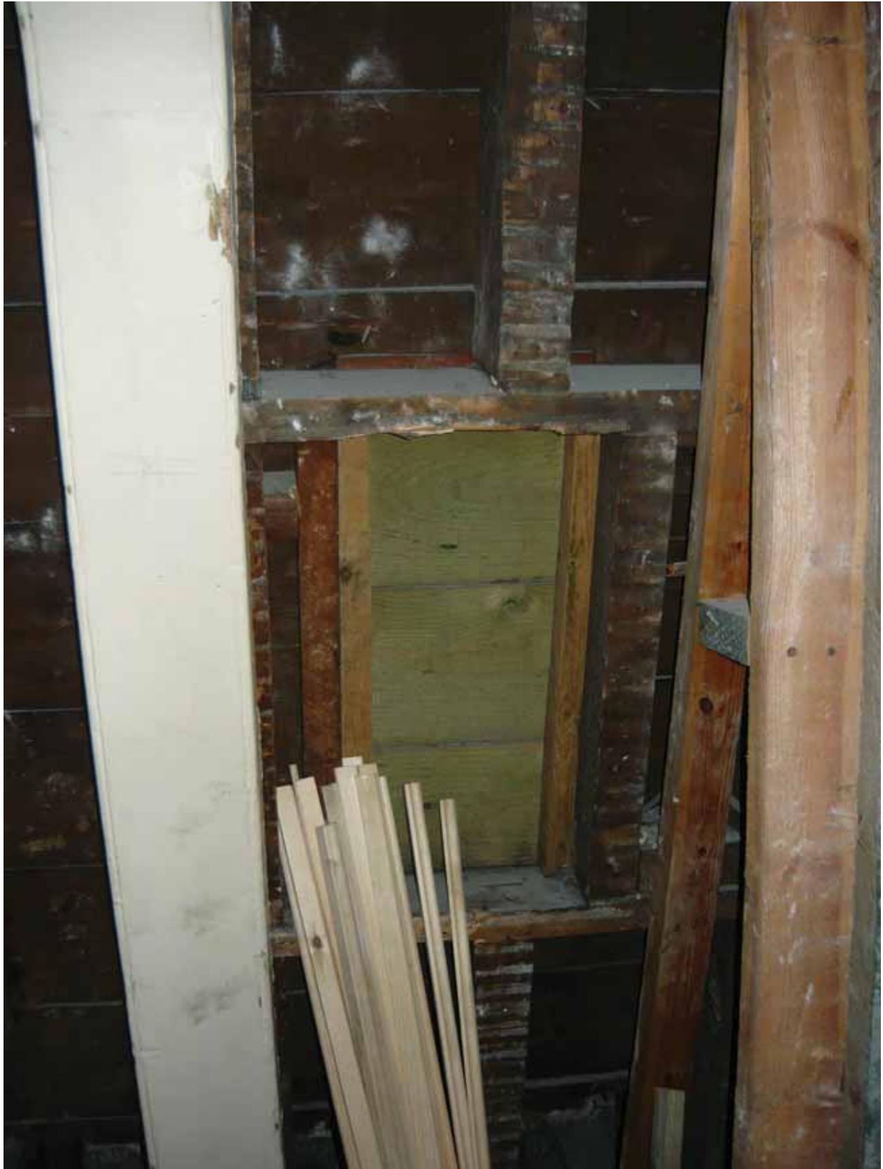
Plate 656: Replaced boards in the roof above Room T120, looking west (EAF10 BHD10 (47))
