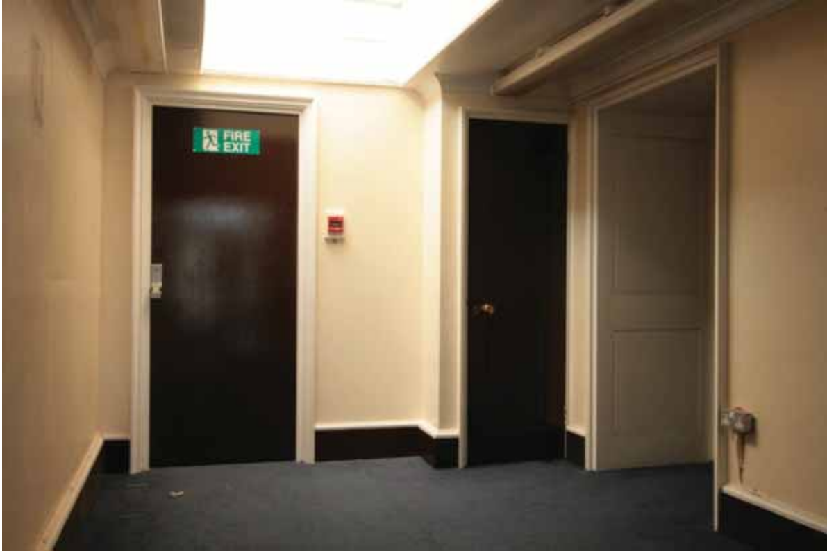
Plate 728: East partition (left), south partition (centre) and west (right) walls in Corridor 10T, looking south (EAF10 57)
