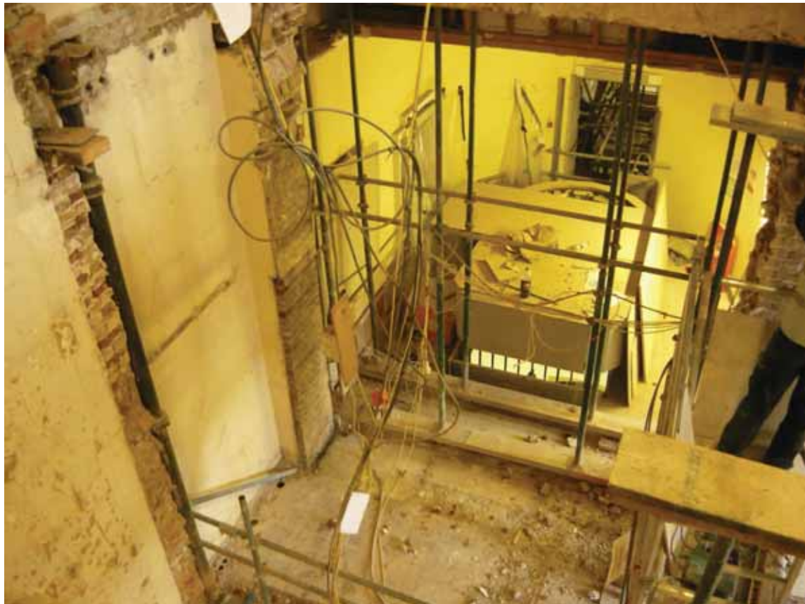
Plate 497b: East (left) wall of Lift/ Cupboard 01F and Corridor 05F and west (right) wall of Corridor 05F, looking south (EAF10 BHD8 (154))
