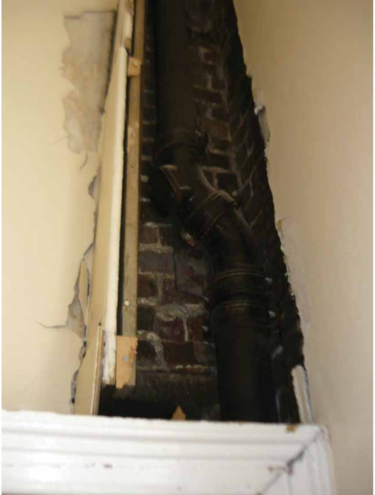
Plate 180: Boxed in pipe in the south-west corner of Room M09, looking south (EAF10 BHD2 (119))
