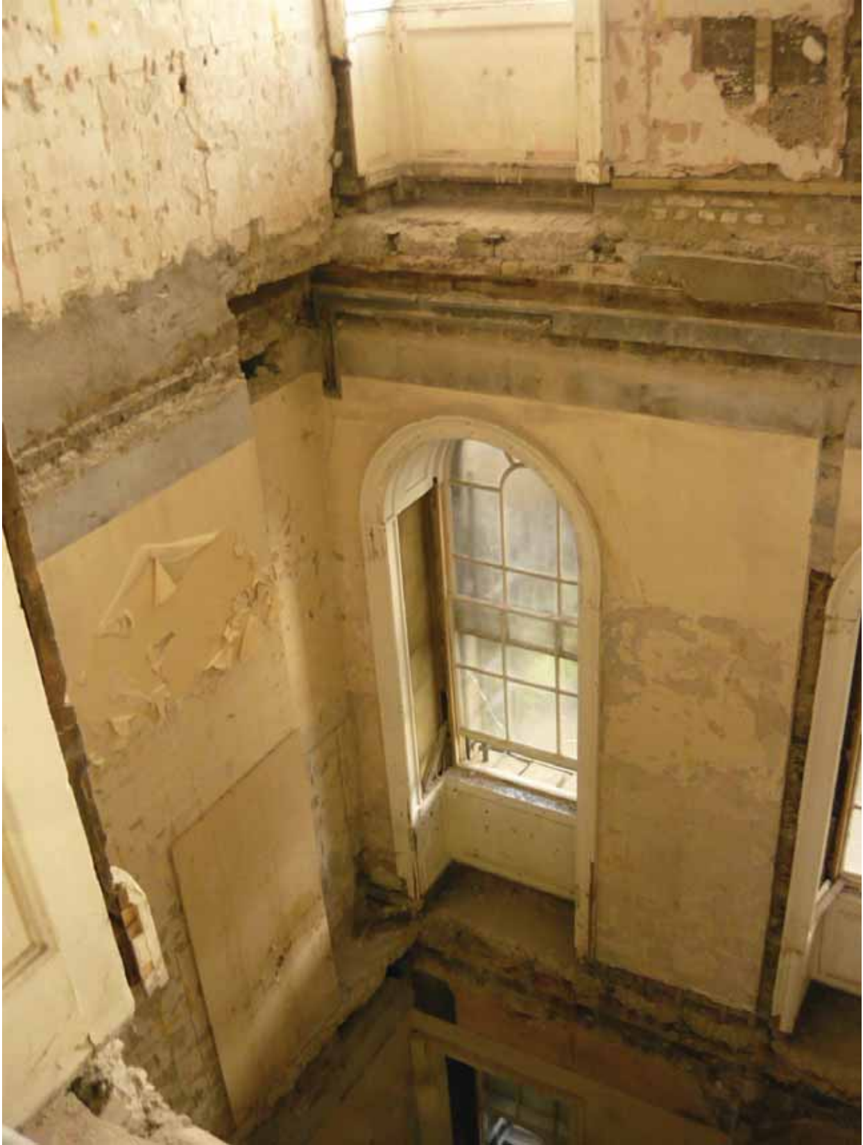
Plate 429: North (left) and east (centre and right) walls in Room G20, looking north-east and down (EAF10 BHD8 (15))
