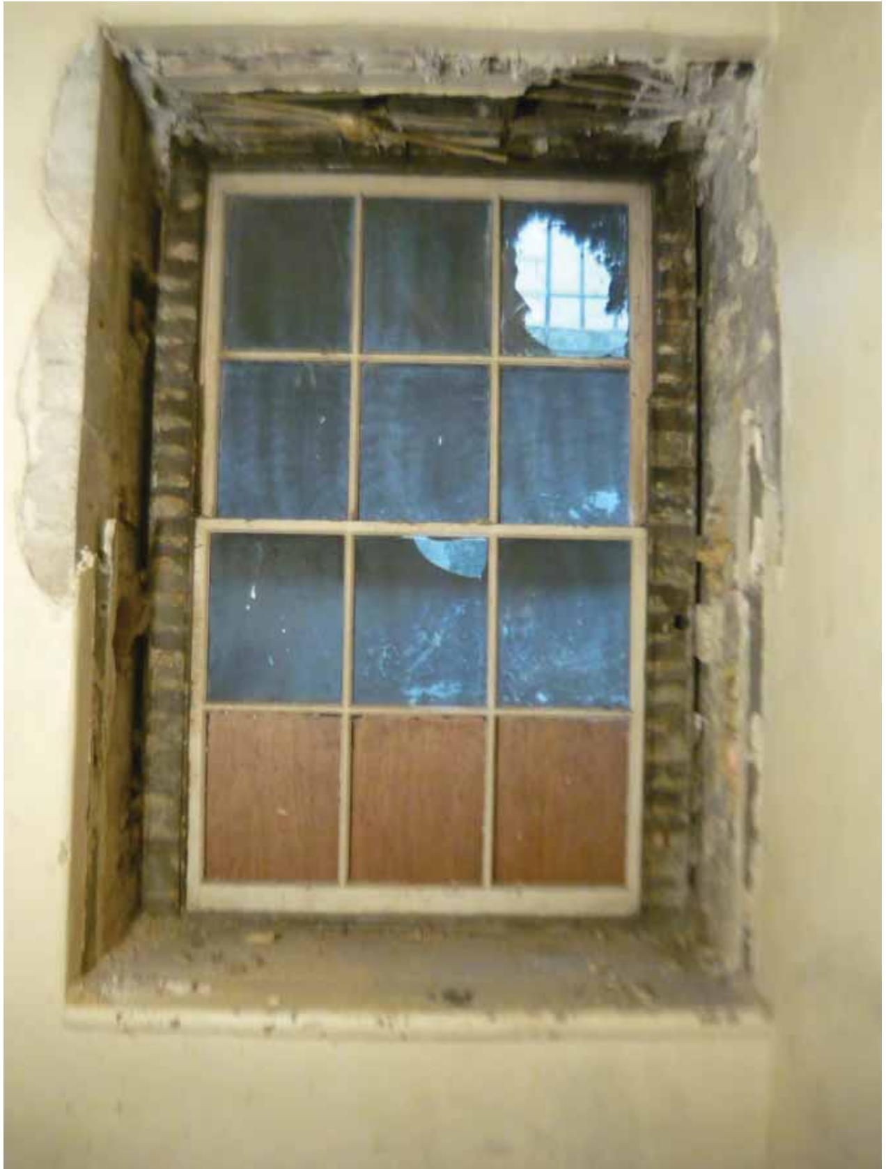
Plate 53a: Sash window in the west wall of Room B48E, looking west (EAF10 BHD5 (53))
