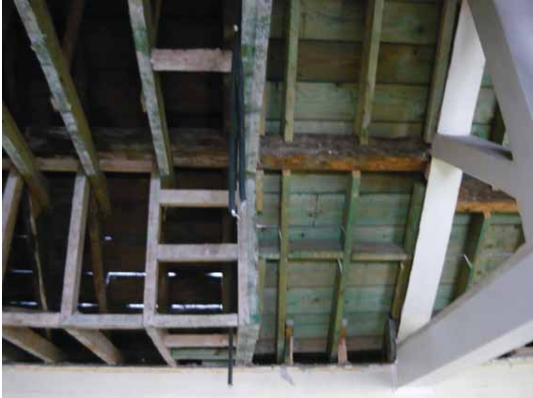
Plate 730: Roof structure above the west wall in Room T115, looking west (EAF10 BHD10 (41))
