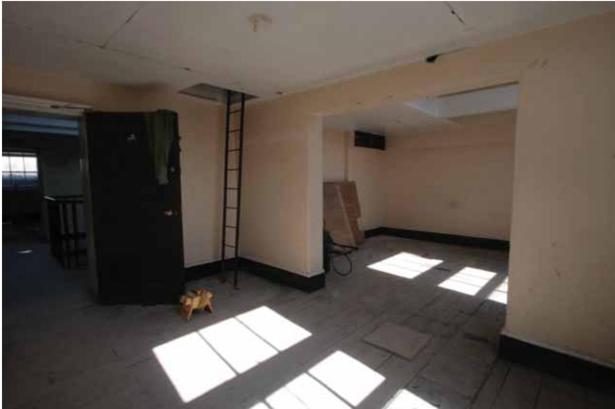
Plate 673: East (left) and south partition (right) walls in Room T04, looking south-west (EAF10 203)
