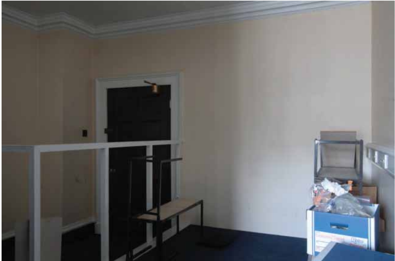
Plate 567: North (left) and east (centre and right) walls in Room S05, looking north-east (EAF10 121)
