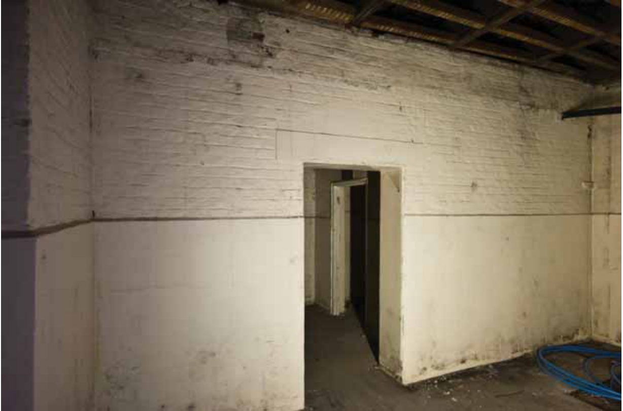
Plate 47: South wall of Room B48A, looking south (DSC_1411 _sitecode EAF10_© PCA Ltd 2010)
