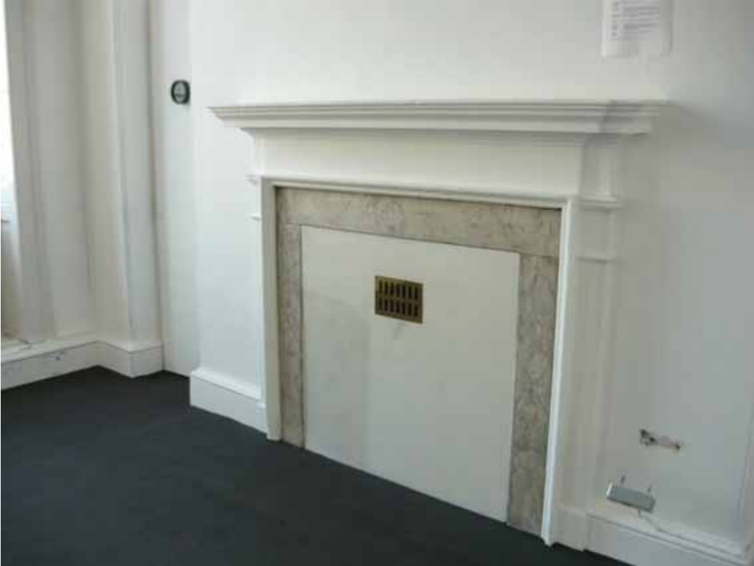
Plate 371: Fireplace (type 6) in the north wall of Room G08, looking north-west (EAF10 BHD1 (39))
