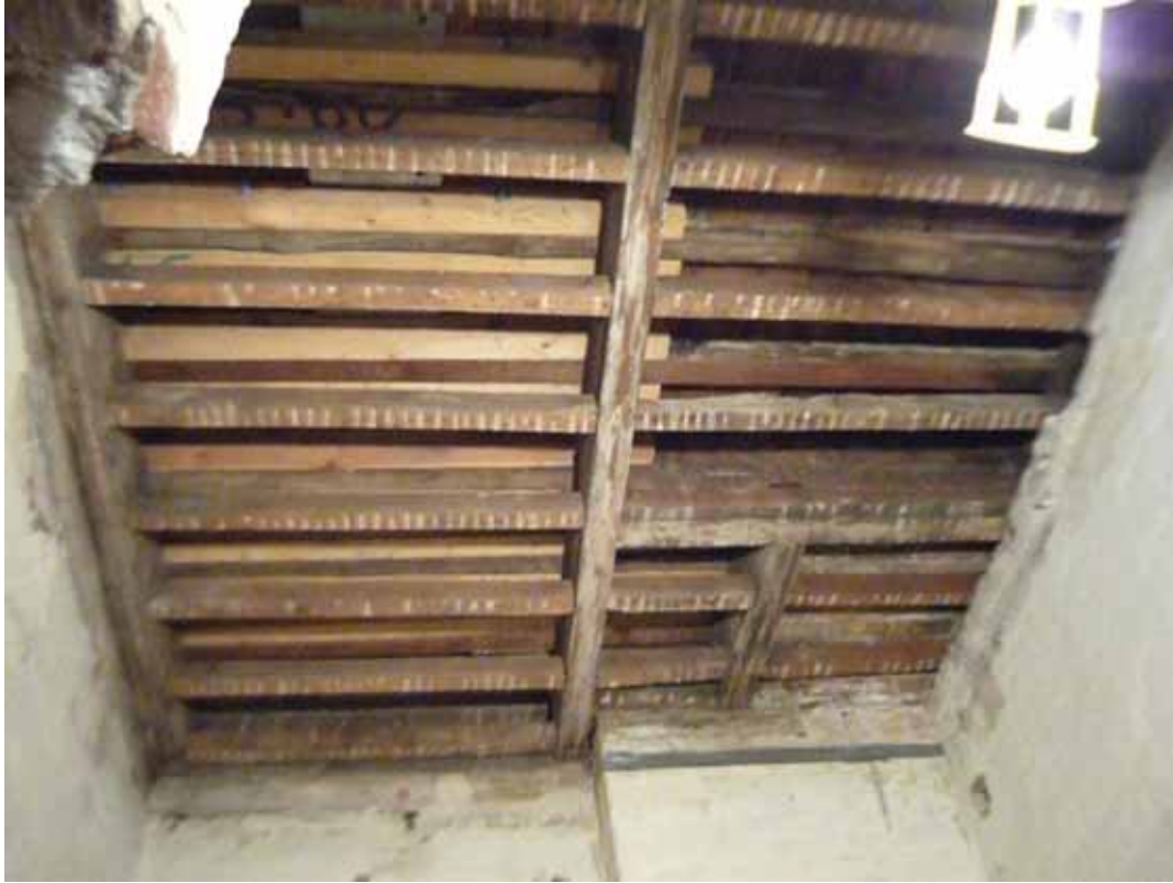
Plate 41: Primary and secondary floor joists visible following the removal of the lath and plaster ceiling in Room B47B, looking south (EAF10 BHD5 (104))
