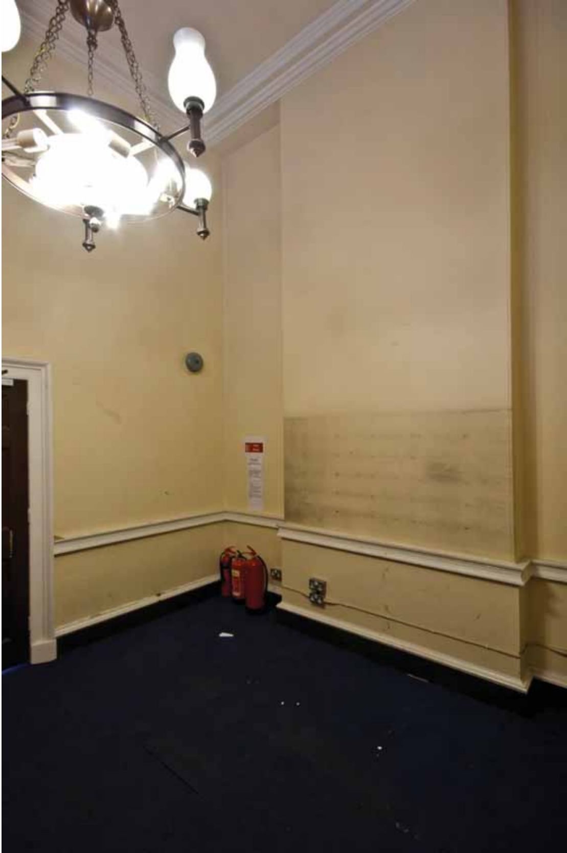
Plate 378: East (left) and south (right) walls in Room G15, looking south-east (EAF10 B100 0946)
