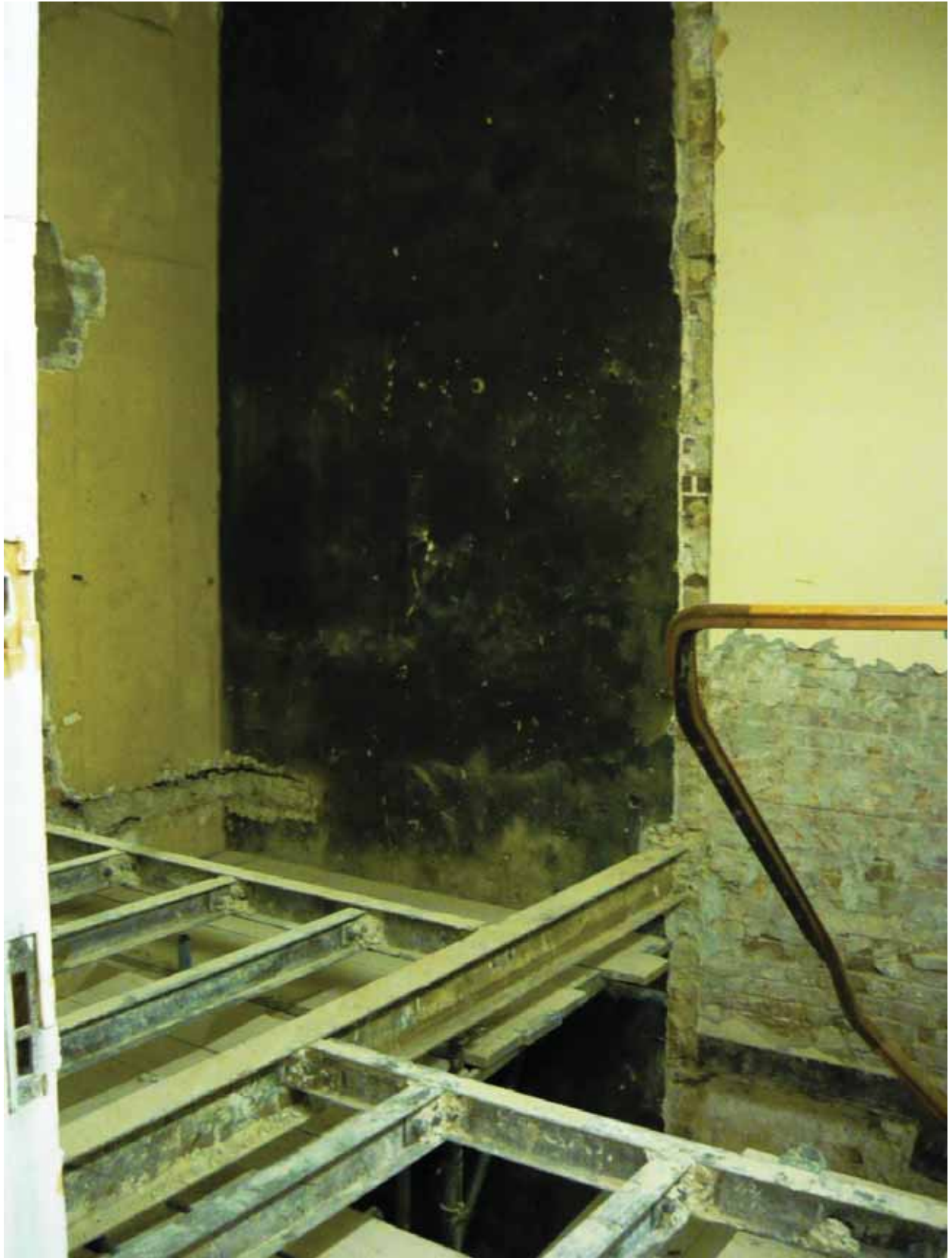
Plate 394: South end of the west wall of Corridor 08G, looking south-west (EAF10 BHD7 (22))
