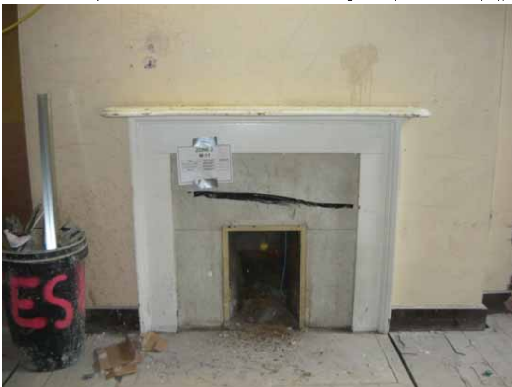
Plate 190: Fireplace in the south wall of Room M11, looking south (EAF10 BHD12 (28))
