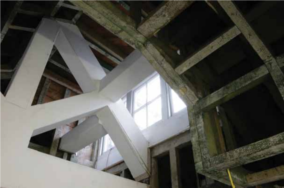
Plate 741: Roof structure above the west wall of Room T118, looking south-west (EAF10 A100 010)
