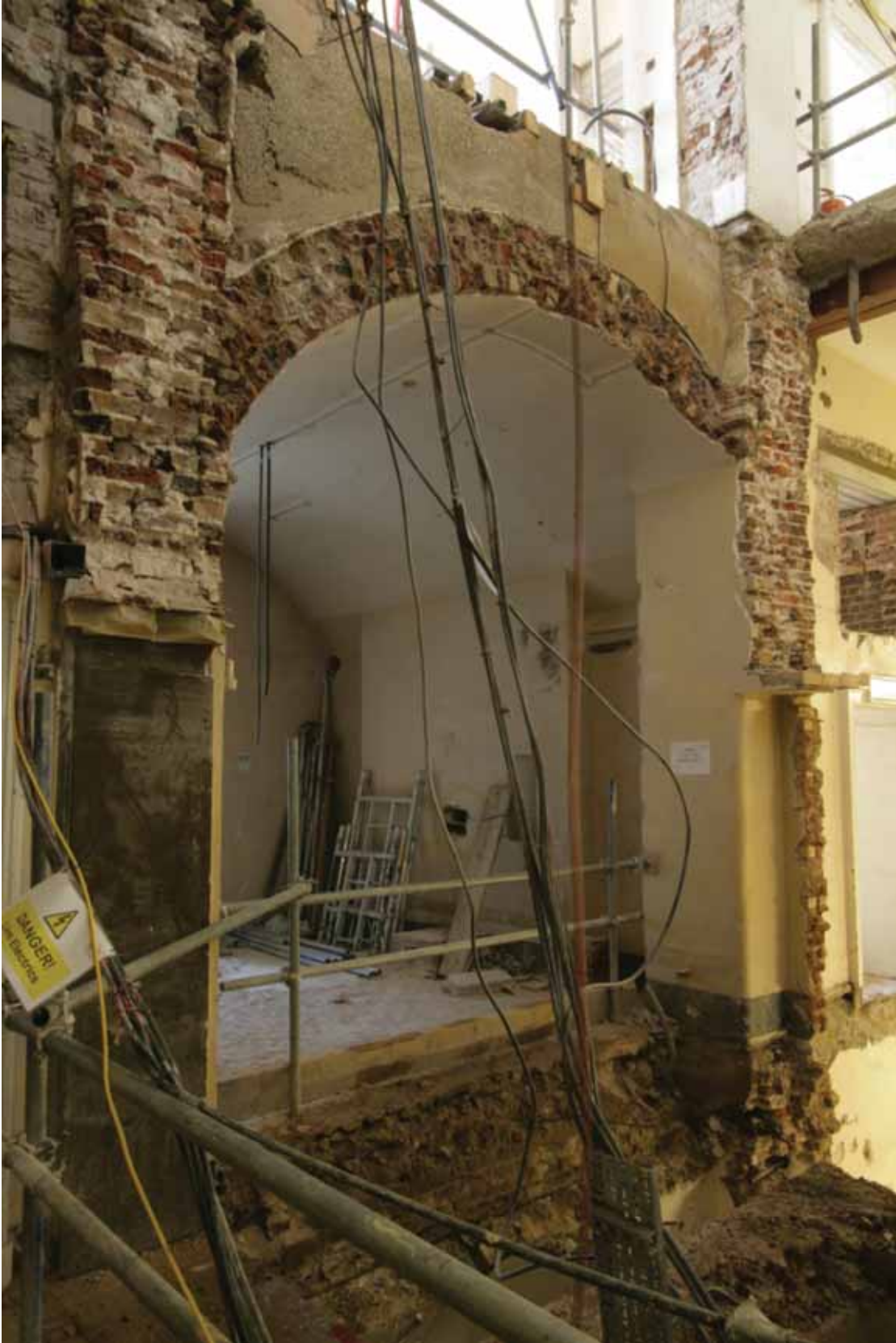
Plate 194a: Brick barrel vaulted ceiling in Room M114, looking north-west (EAF10 A-D101 004)
