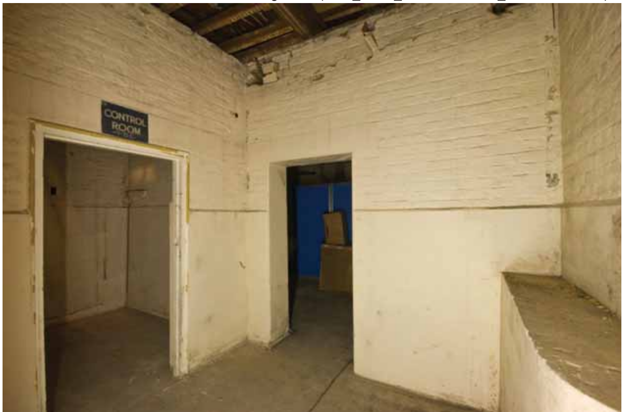
Plate 48: West (left) and north (right) walls of Room B48B, looking north –west (DSC_1416 _sitecode EAF10_© PCA Ltd 2010)
