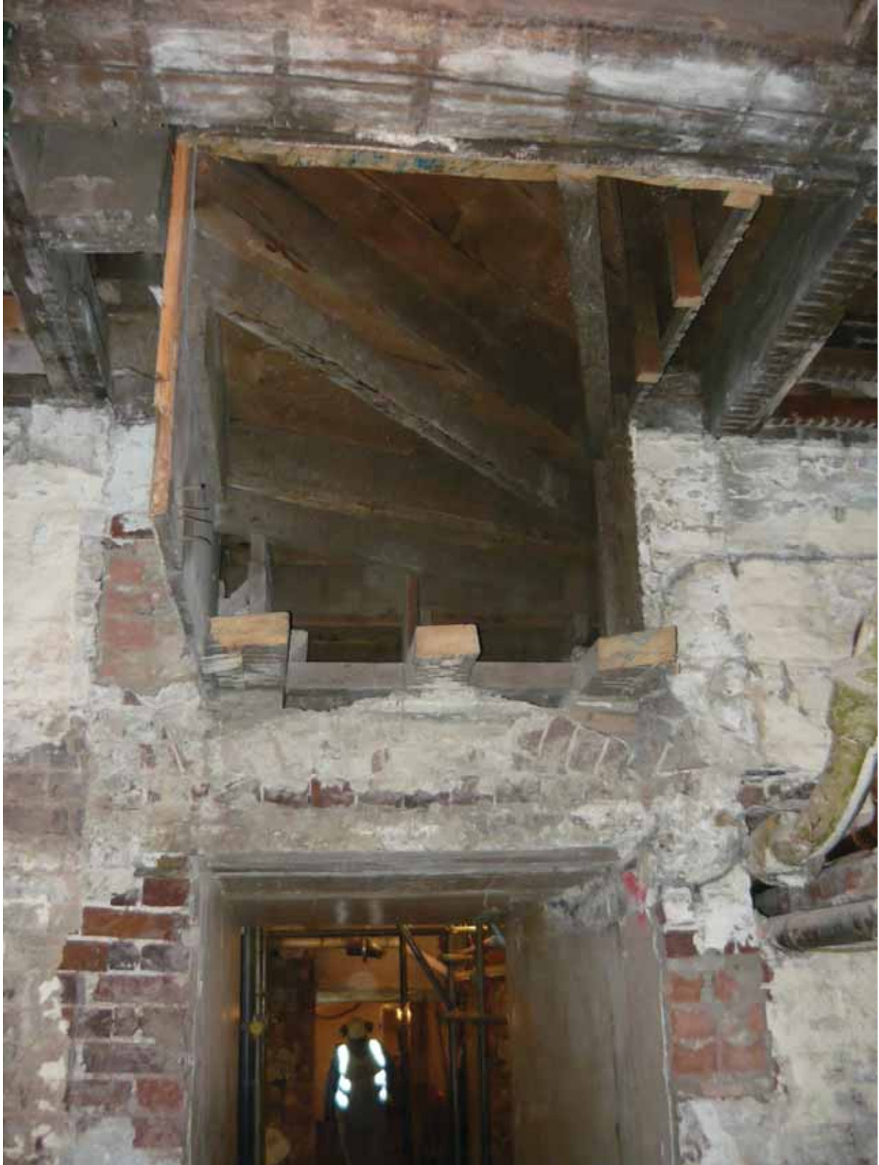
Plate 70: South doorway in Room B63 following removal of its concrete surround, looking south (EAF10 BHD6(36))
