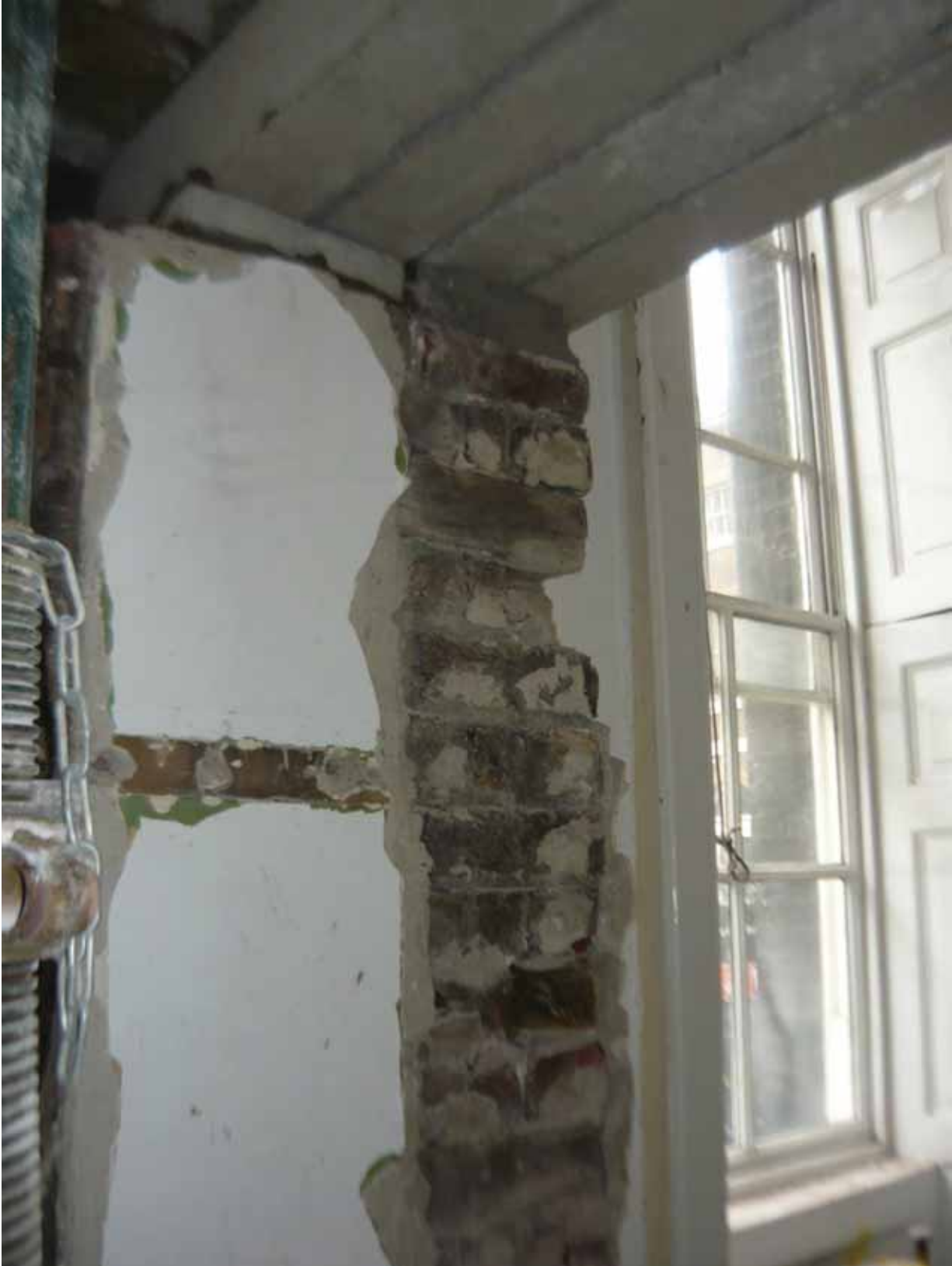
Plate 411: Doorway opened up at the east end of the south wall in Room G16, looking south-east (EAF10 BHD3 (39))
