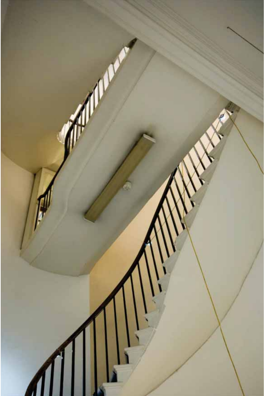
Plate 502: Underside of link bridge in Stairs 02F, looking up and north-west (EAF10 B100 0845)
