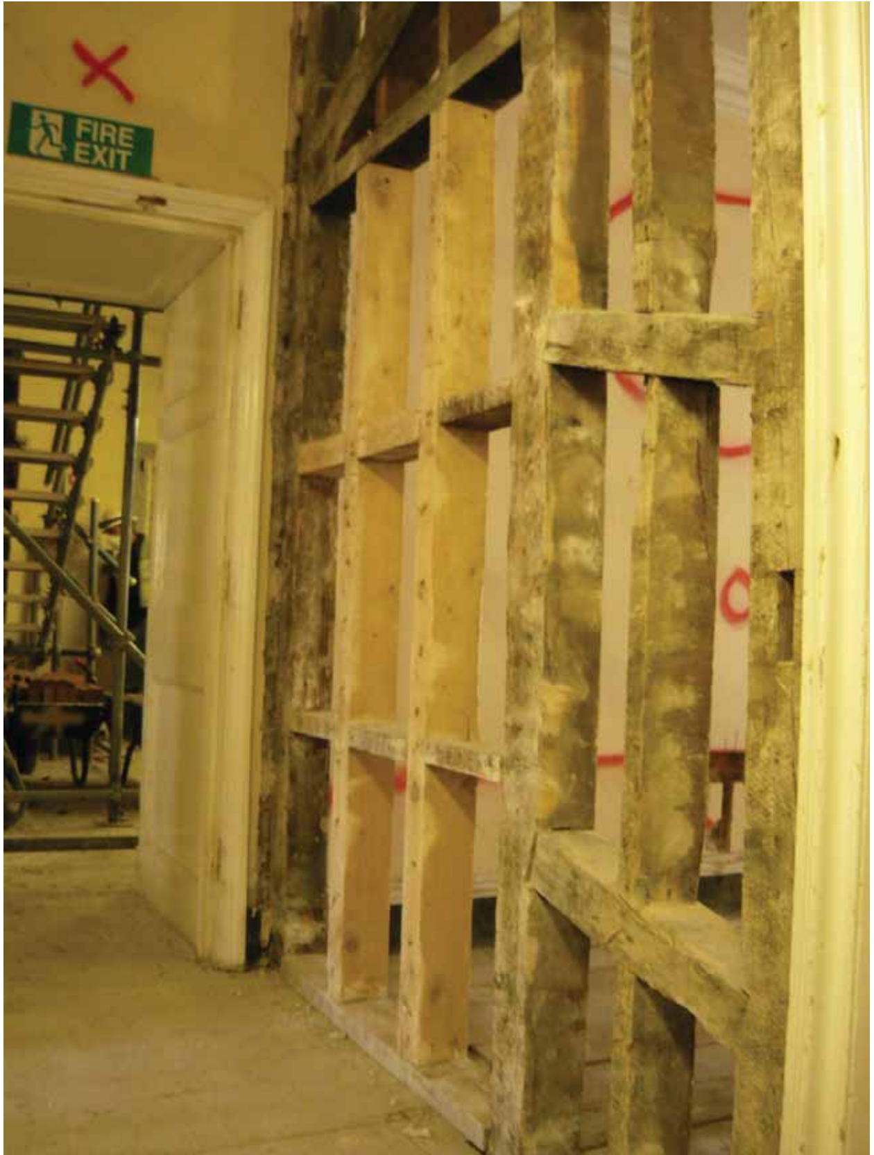
Plate 617: North (left) and east partition (right) walls in Room S16, looking north-east (EAF10 BHD8 (36))
