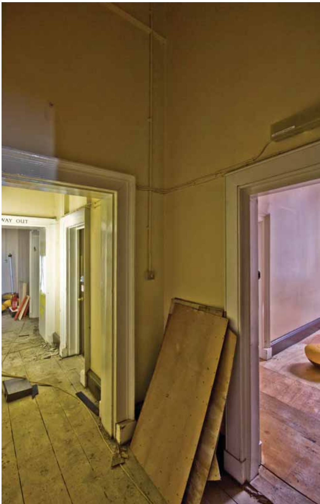
Plate 301: East partition wall in north-south corridor through Room M26/M27, looking north-east (EAF10 LG100 1019)
