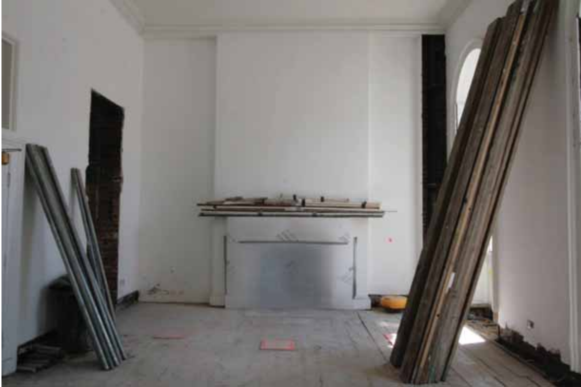
Plate 369: East (left), south (centre) and west (right) walls in Room G08, looking south (EAF10 267)
