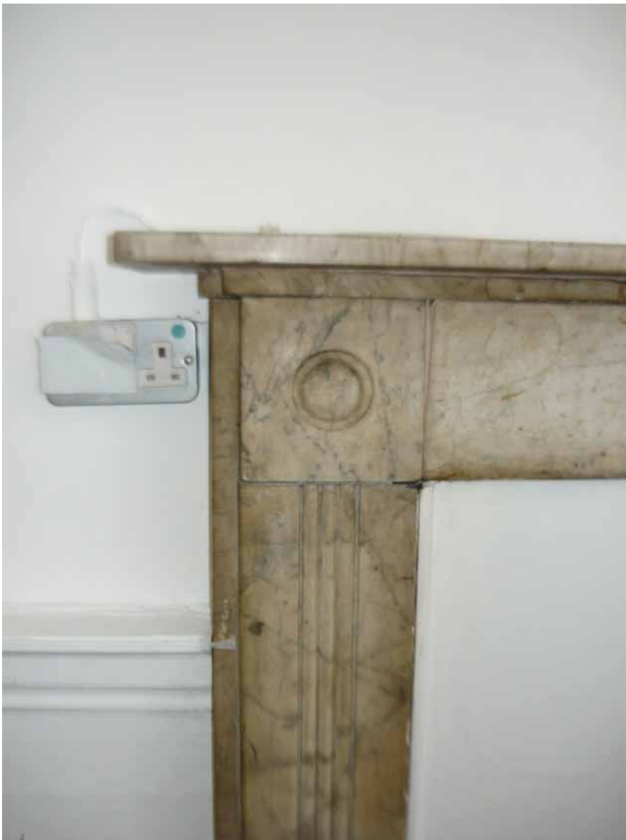
Plate 414: West side of the fireplace (type 21) in the north wall of Room G17, looking north (EAF10 BHD1 (56))
