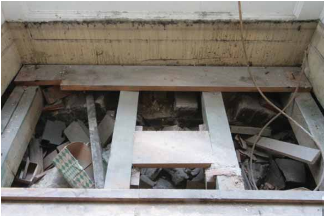
Plate 308: Remains of a brick segmental arch under the south window in the east wall of Room M26/M27, looking east (EAF10 298)
