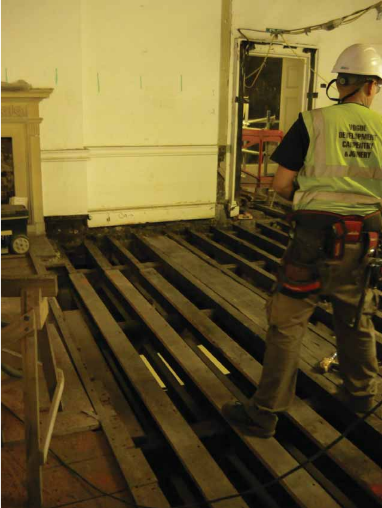
Plate 410: South wall of Room G16 (left of partion scar) and Corridor 07G (right of partion scar) looking south (EAF10 BHD8 (121))
