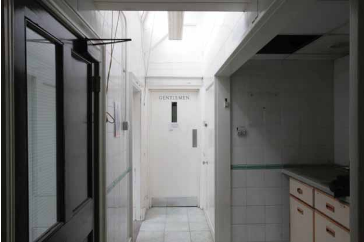
Plate 755: West (left), north (centre) and east partition (right) walls in Room T20, looking north (EAF10 40)
