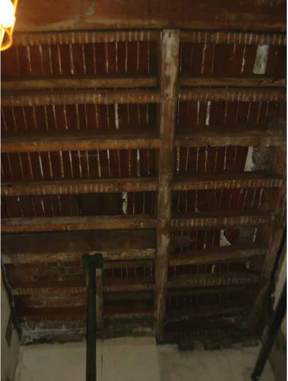
Plate 24a: Primary and secondary floor joists visible following the removal of the lath and plaster ceiling in Room B46, looking south (EAF10 BHD5 (201))
