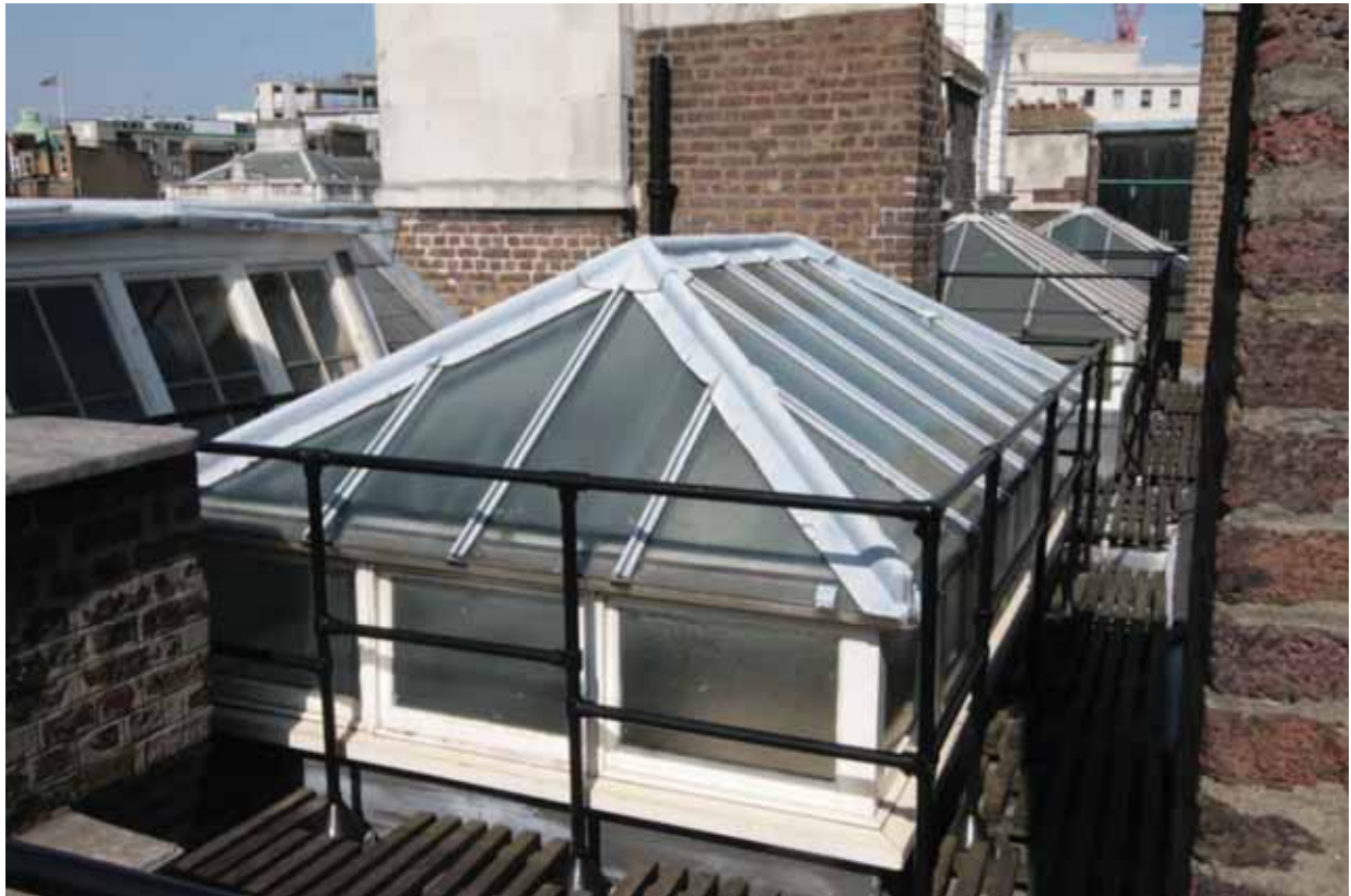
Plate 796: Lantern skylight over the west end of Room T15, looking north-west (EAF10 25)
