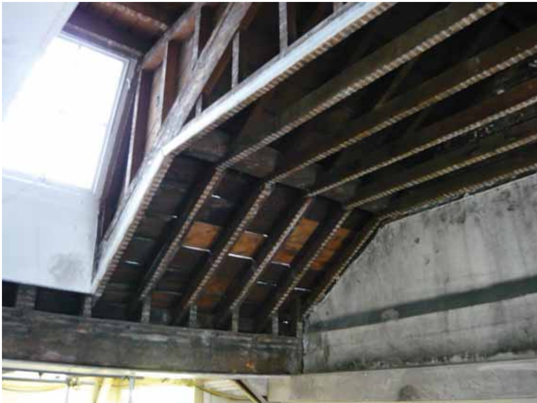
Plate 748: North end of the west side of the roof above Room T15, looking west (EAF10 BHD10 (29))
