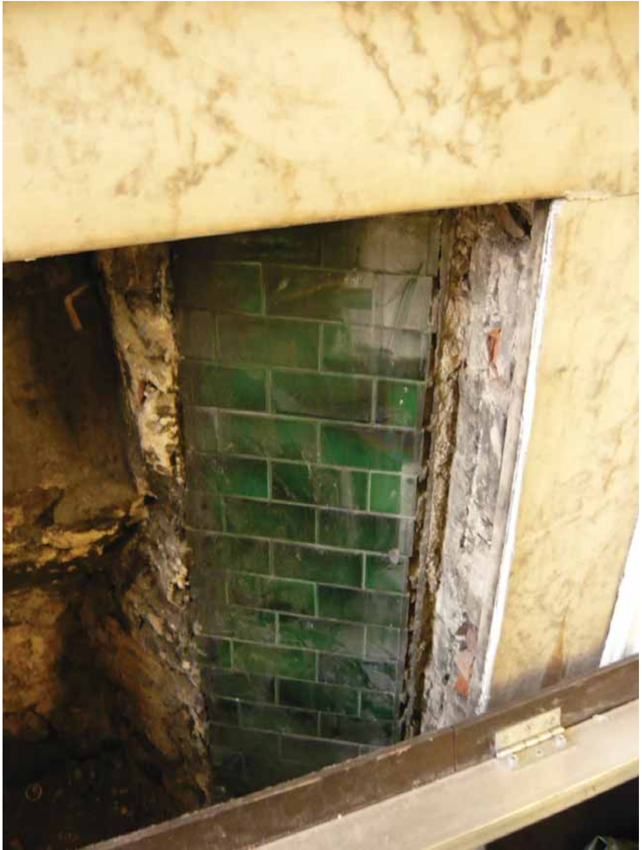
Plate 479: East side of the fireplace in the north wall of Room F05, looking north-east (EAF10 BHD8 (13))
