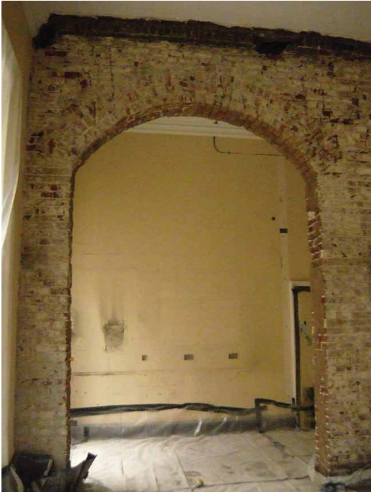
Plate 319: Arch in south partition wall in Room M29a, looking south (EAF10 BHD6 (14))
