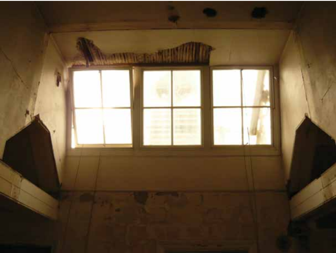
Plate 760: West (left and centre) and north(right) walls in Room T20, looking west (EAF10 195)
