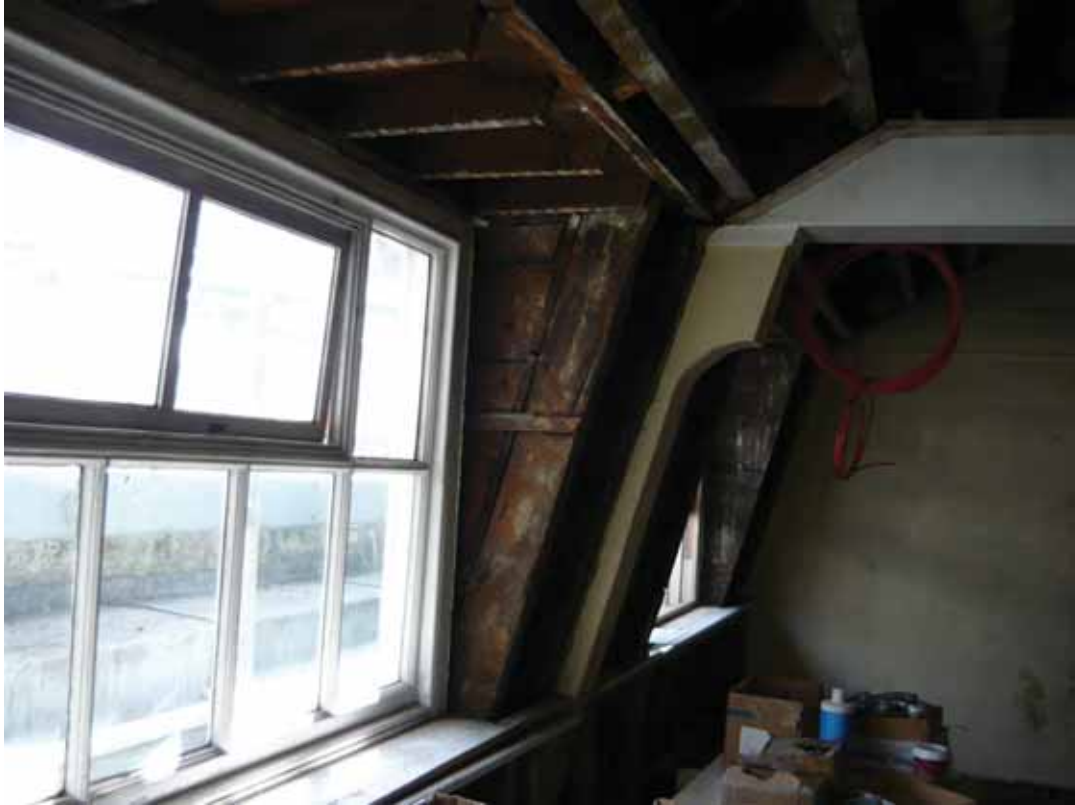
Plate 734: East (left) and south (right) walls in Room T117, looking south-east (EAF10 BHD10 (35))
