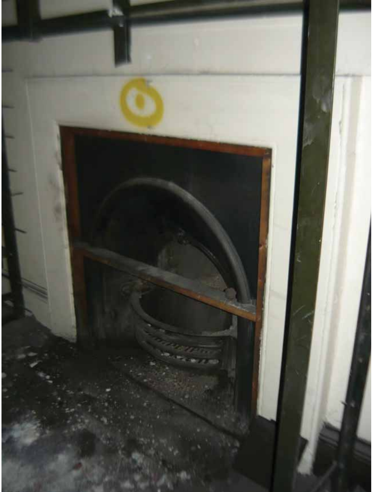
Plate 313: Fireplace in the south wall in Room M28, looking south-east (EAF10 BHD3 (99))
