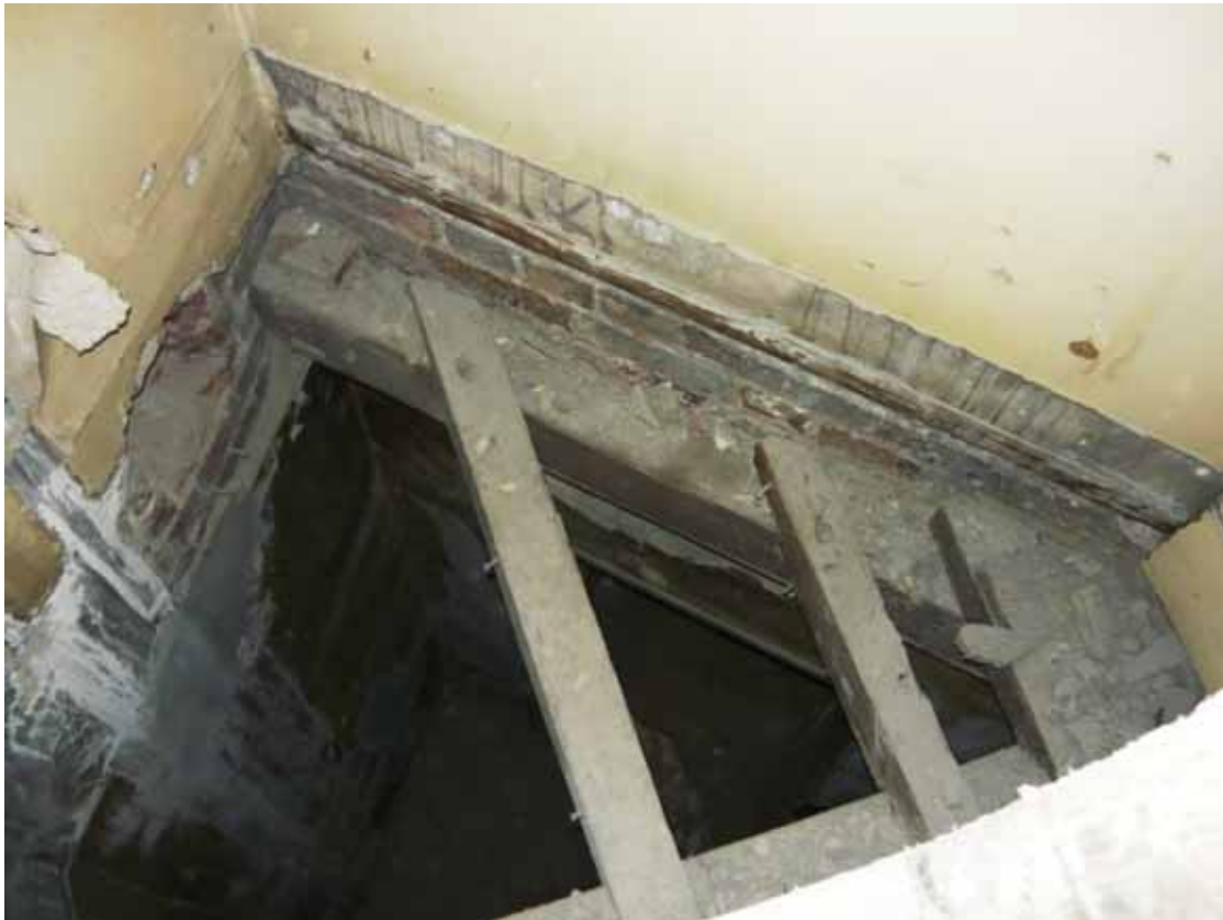
Plate 357: Inside cupboard at the south end of the east wall in Room G03, looking down and east (EAF10 BHD7 (25))
