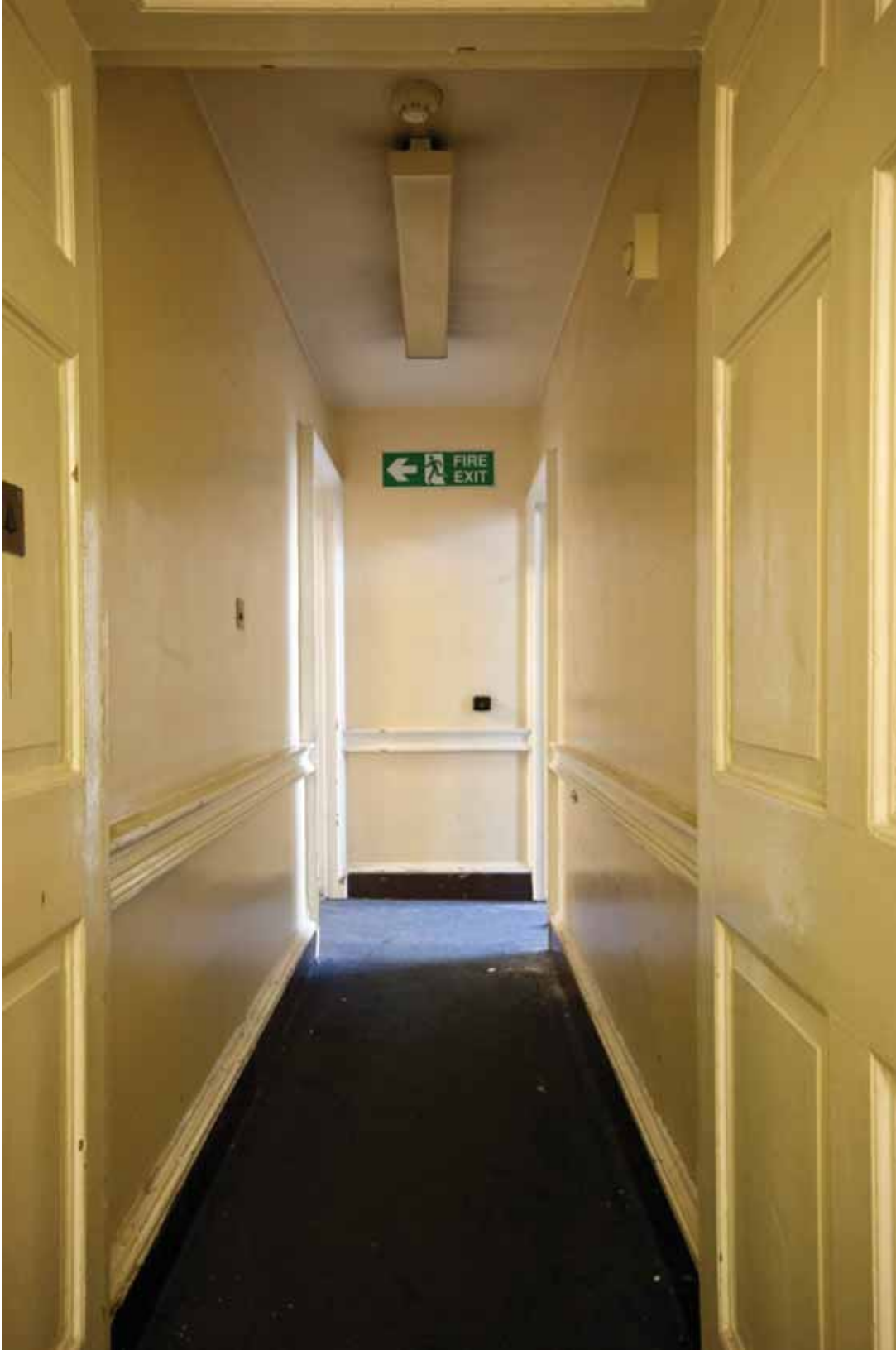
Plate 447: West (left), north (centre) and east partition (right) walls in Room G28, looking north (EAF10 B100 0928)
