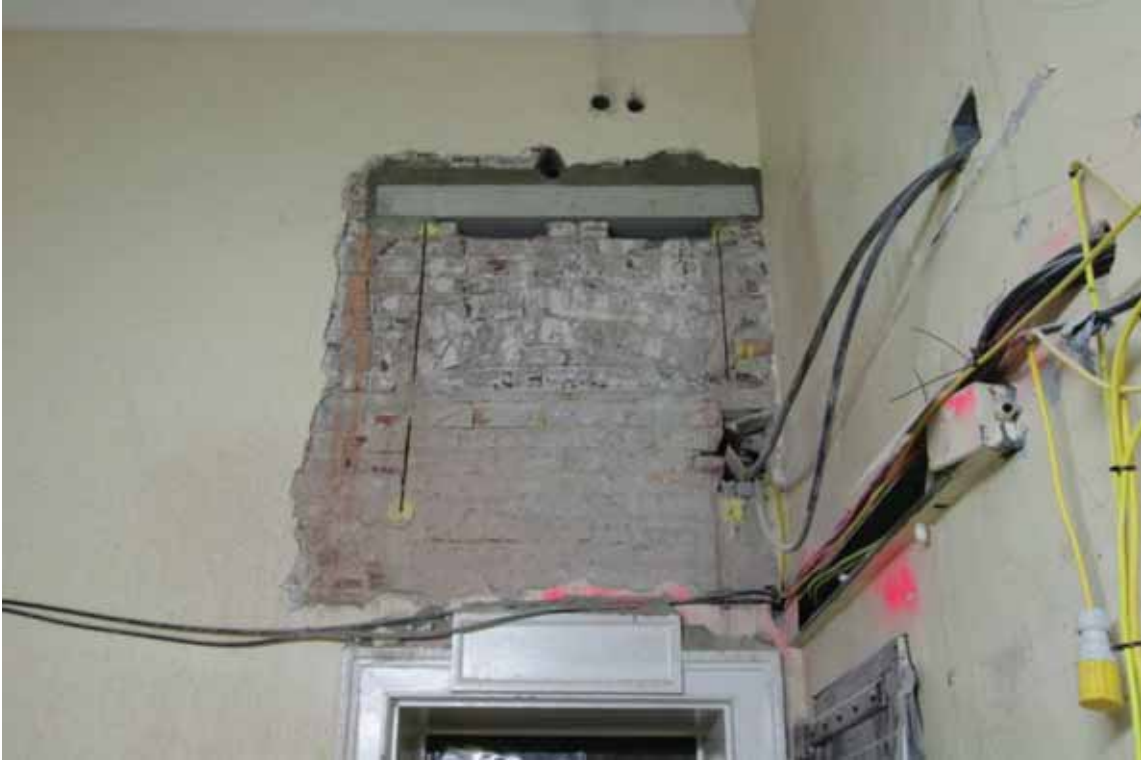
Plate 234: Infilled fan light over the doorway at the north end of the west wall of Corridor 04LG, looking west (EAF10 A100 029a)
