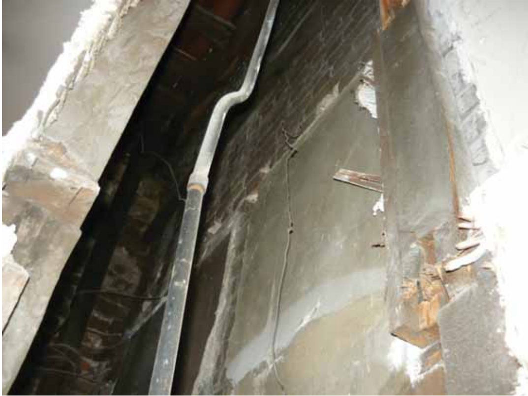
Plate 525: Void at the north end of the partition wall in Room F16, looking up and north-west (EAF10 BHD8 (30))
