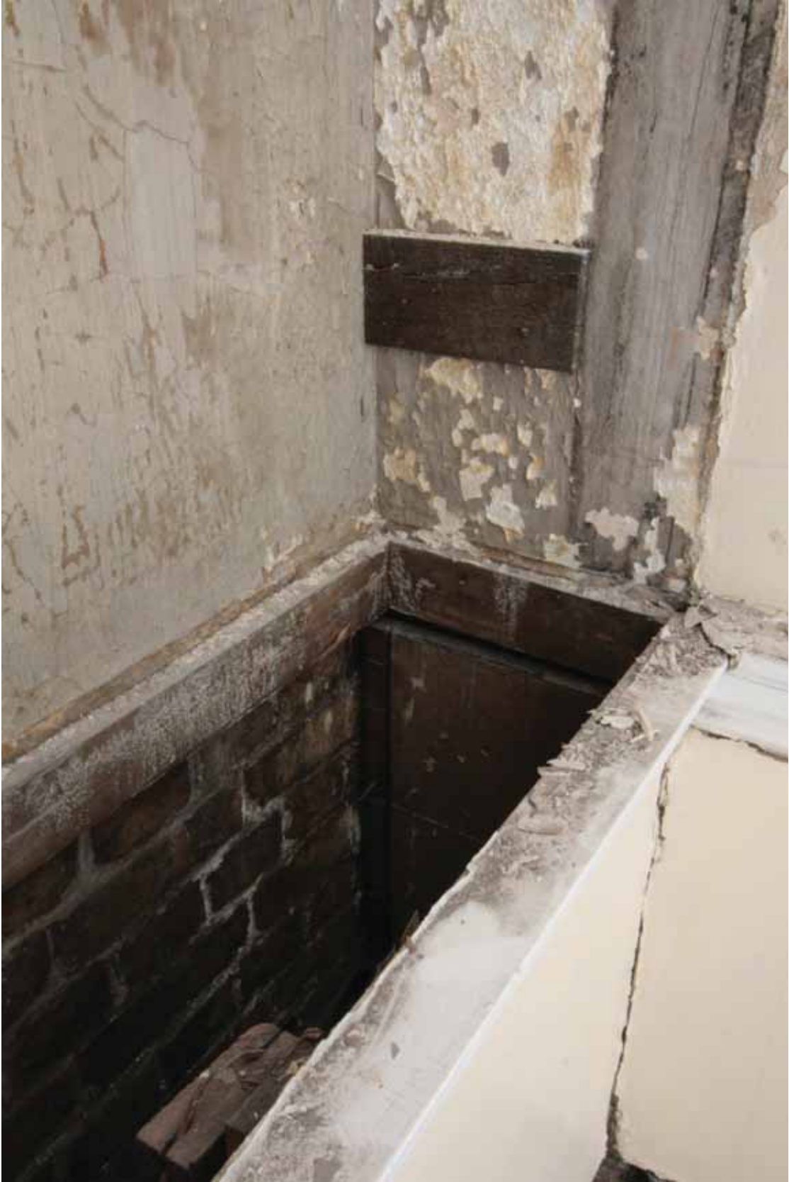
Plate 469: West end of the south wall in Room F03, looking south-west (EAF10 243)
