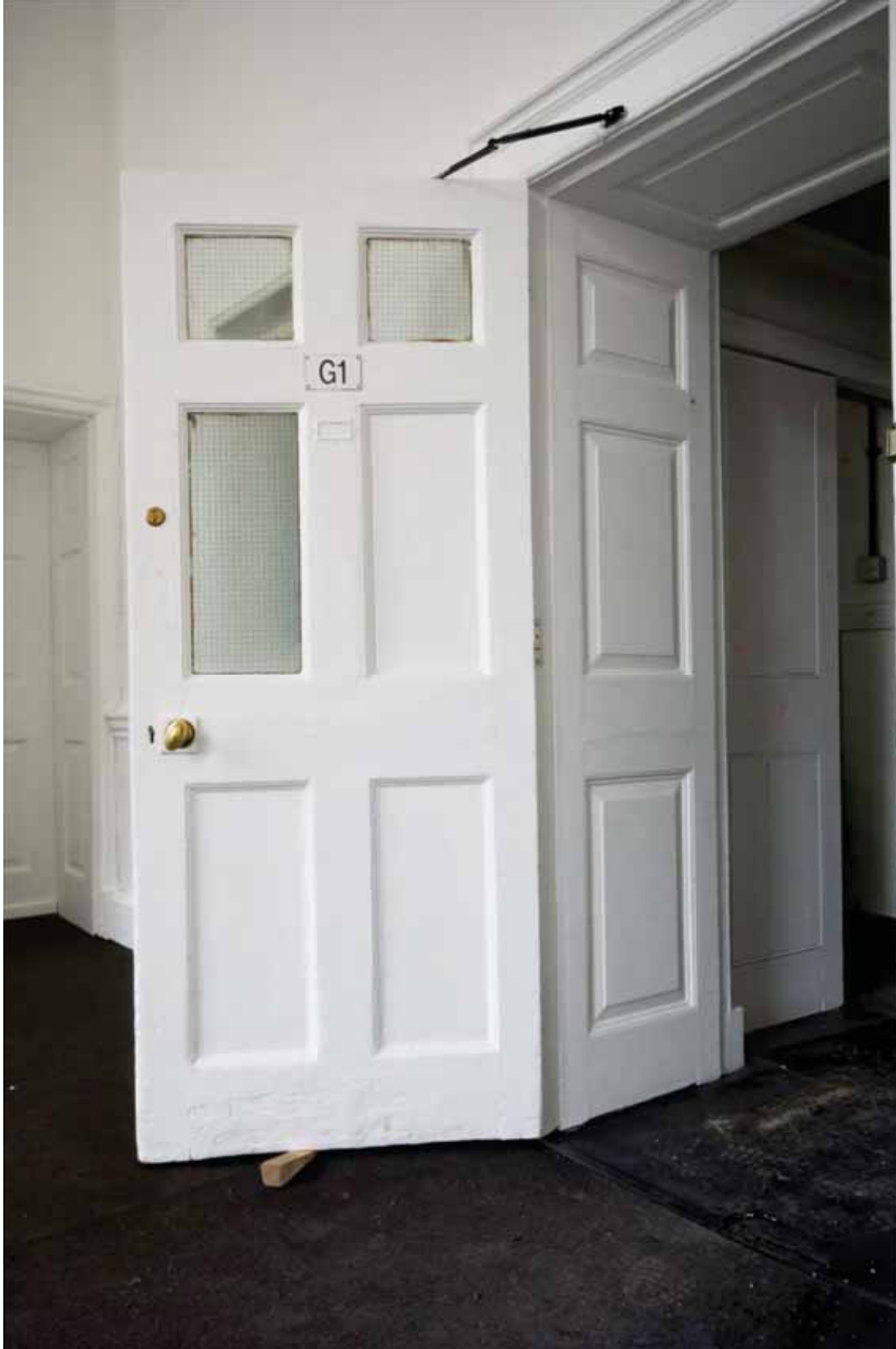
Plate 345: Doorway (type 41) in the east wall of Room G01, looking north-east (DSC_0834 sitecode EAF10 © PCA Ltd 2010)
