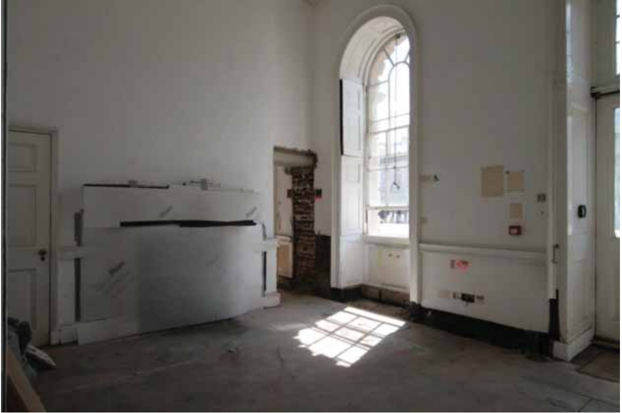
Plate 364: South (left) and west (right) walls in Room G06, looking south-west (EAF10 271)
