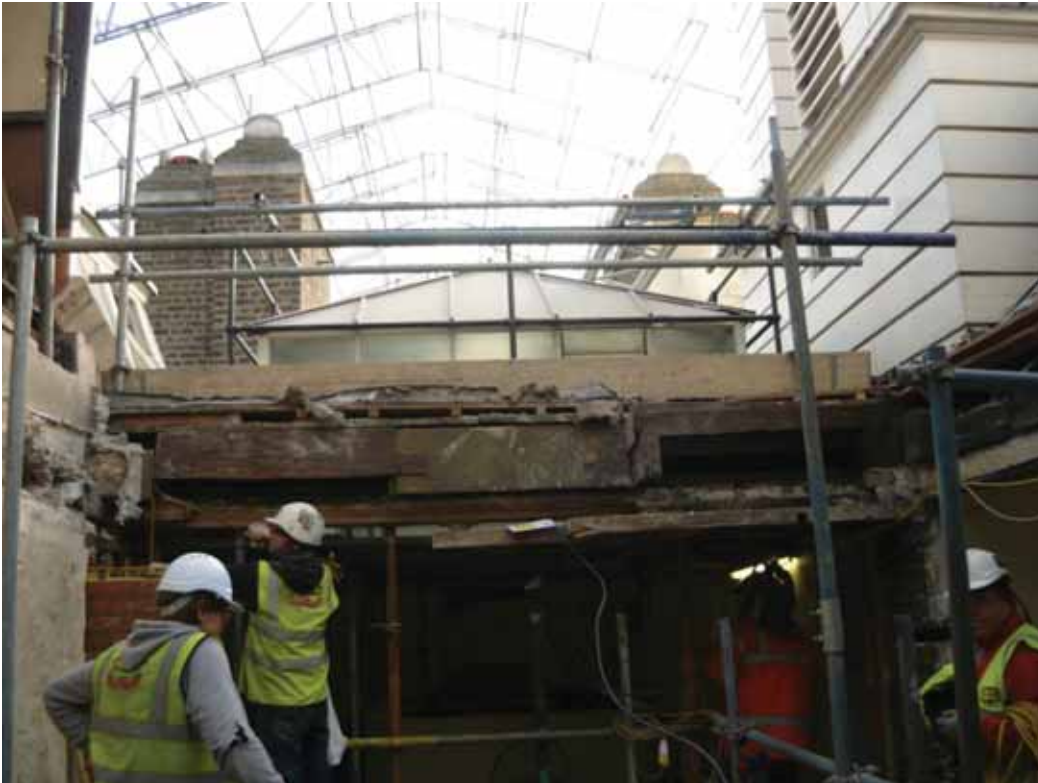
Plate 809: Lantern skylight over Corridor 05T and removed south wall of Cupboard 01T and Corridor 04T, looking south (EAF10 BHD8 (52))
