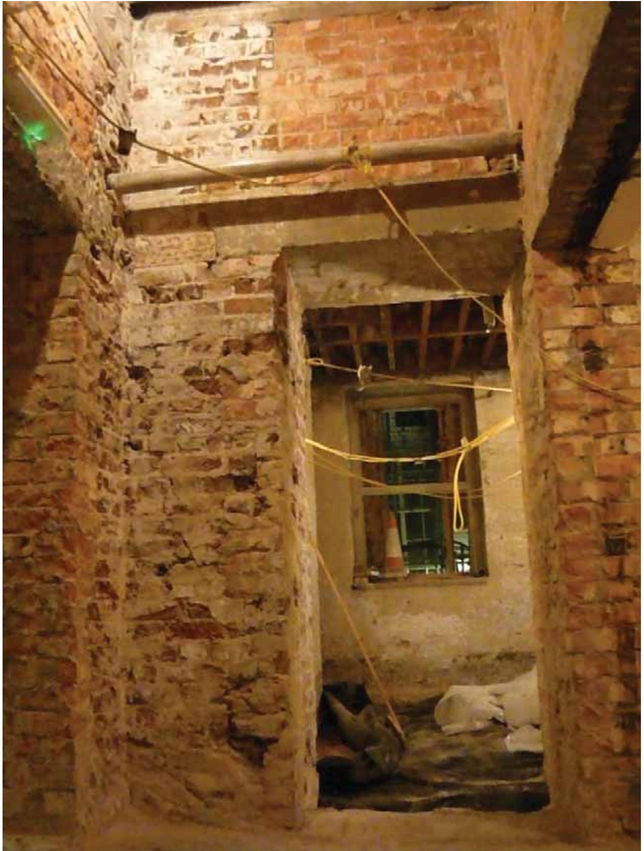
Plate 79: East wall of Corridor 1A, looking east into Room B51 (EAF10 BDH6(61))
