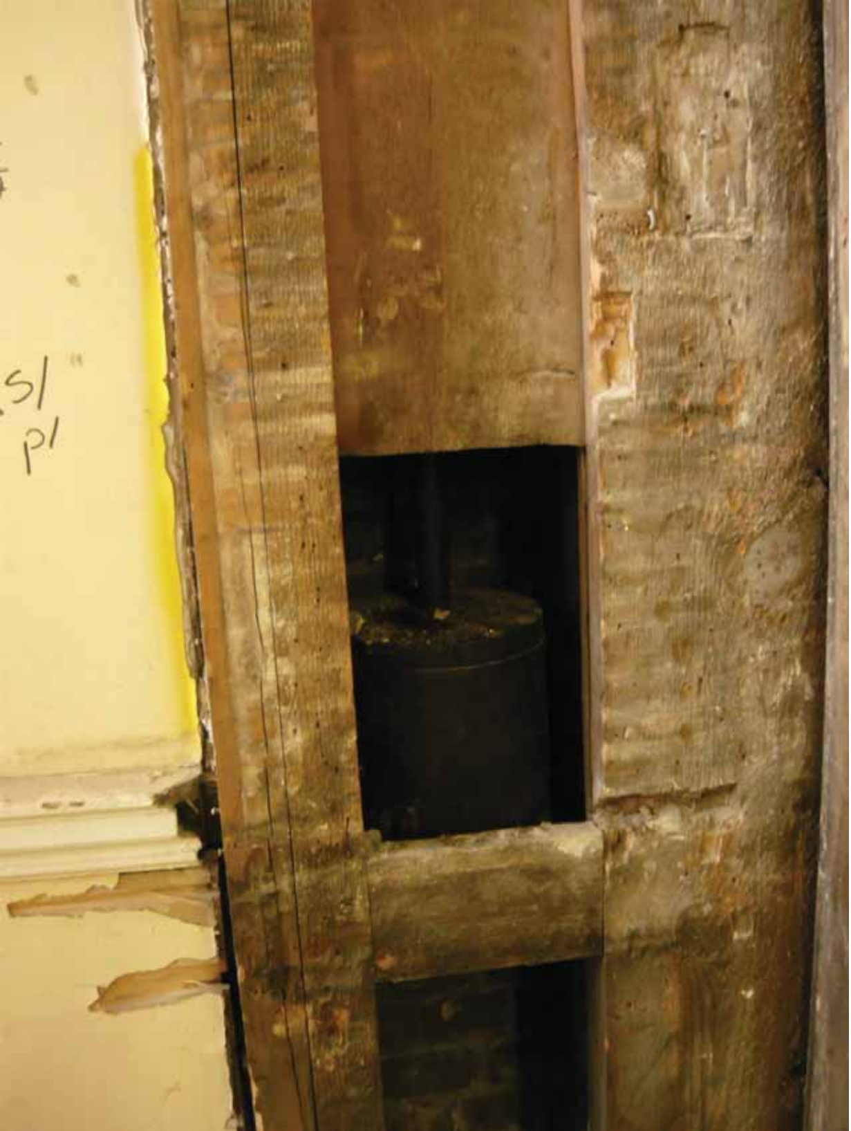
Plate 475: Boxed in weight for the clock in the north-east corner of Room F03, looking north (EAF10 BHD8 (18))
