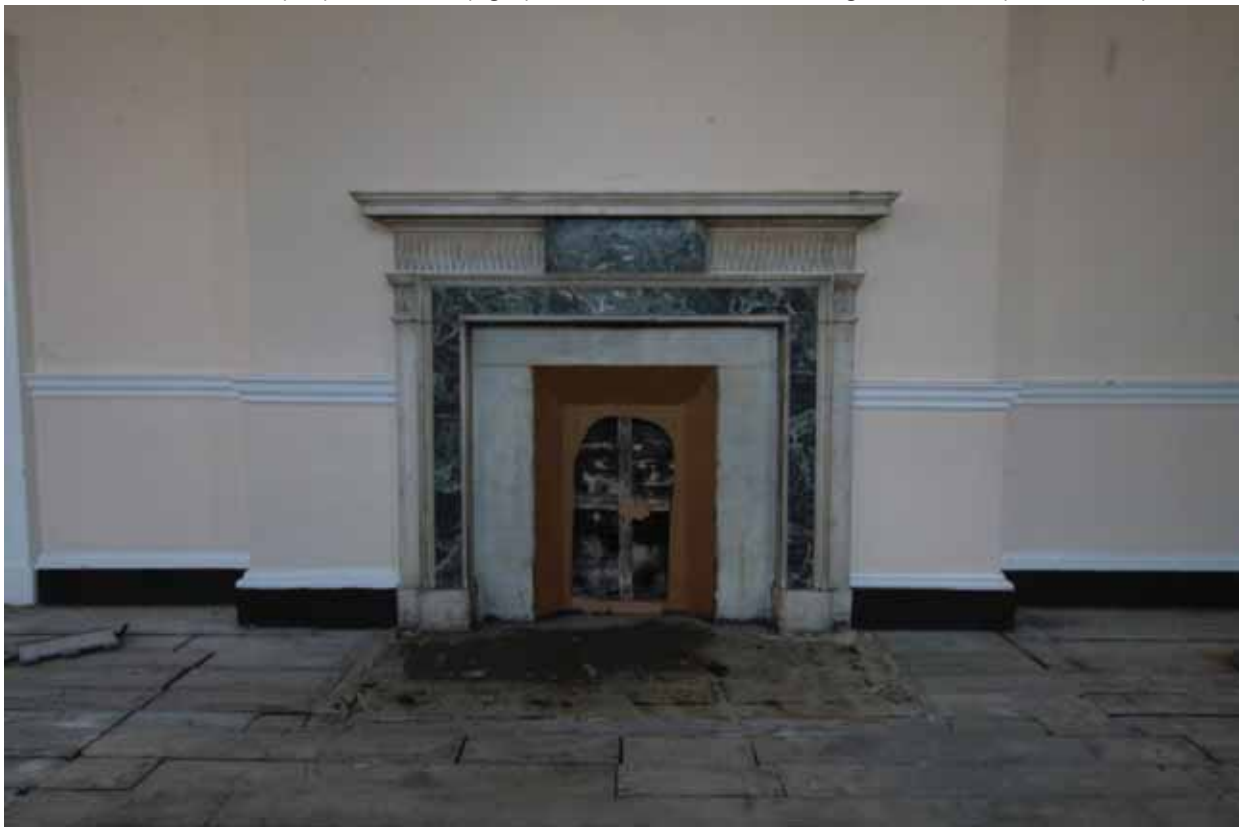
Plate 484: Fireplace (type 13) in the east wall of Room F09, looking east (EAF10 146)
