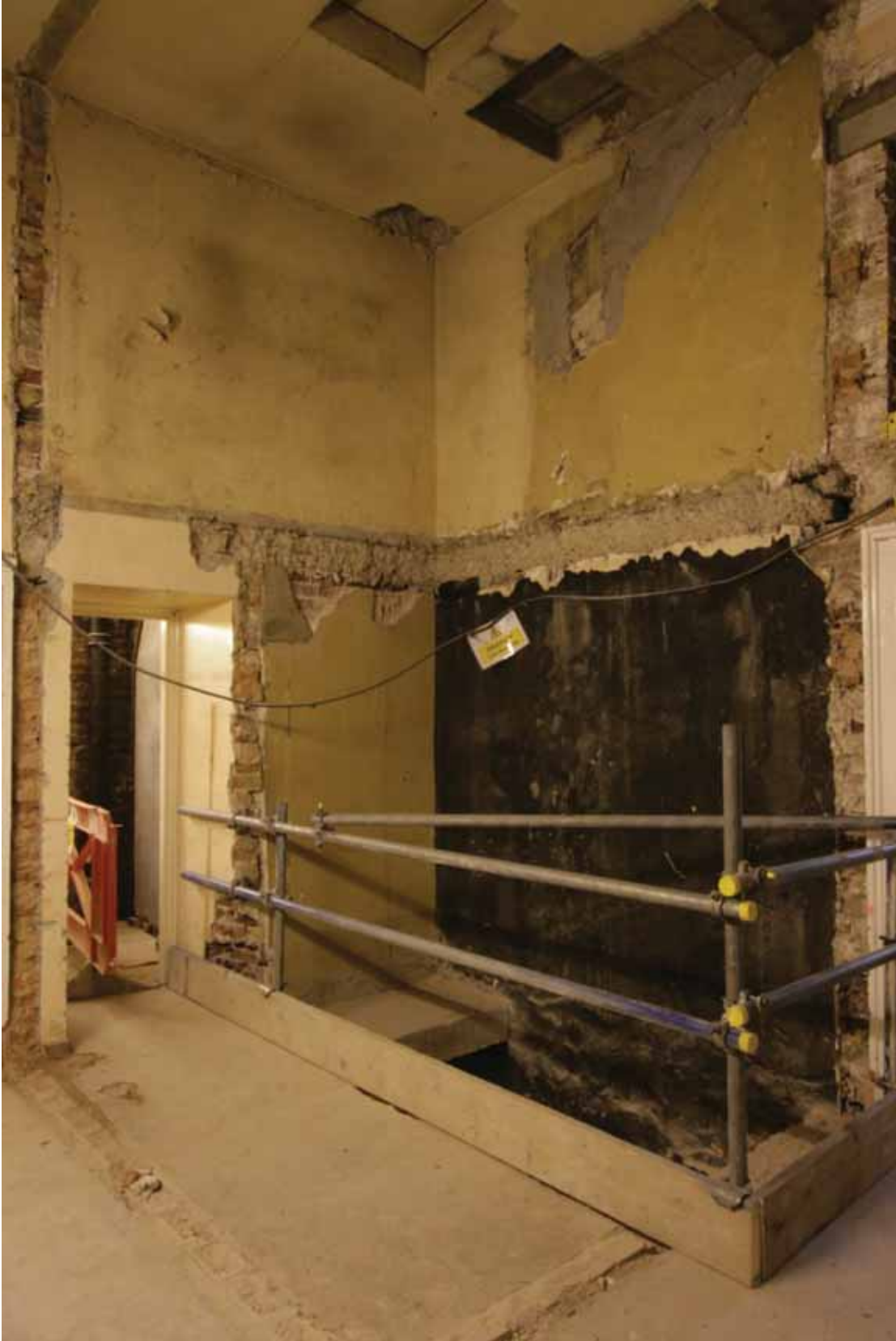
Plate 507: South (right) and west walls in Corridor 07F following the removal of the dumb waiter, looking south-west (EAF10 A100 022)
