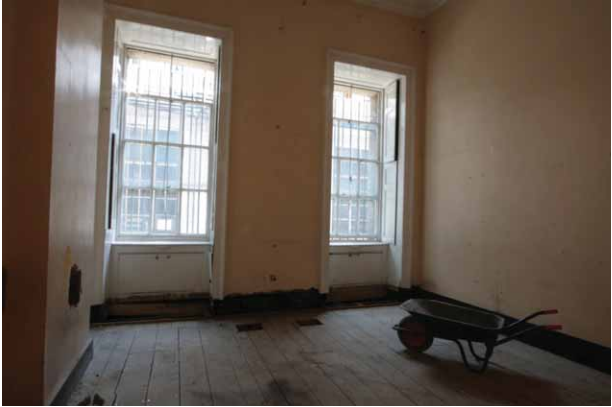
Plate 297: Two windows in the east wall of Room M25, looking east (EAF10 296)
