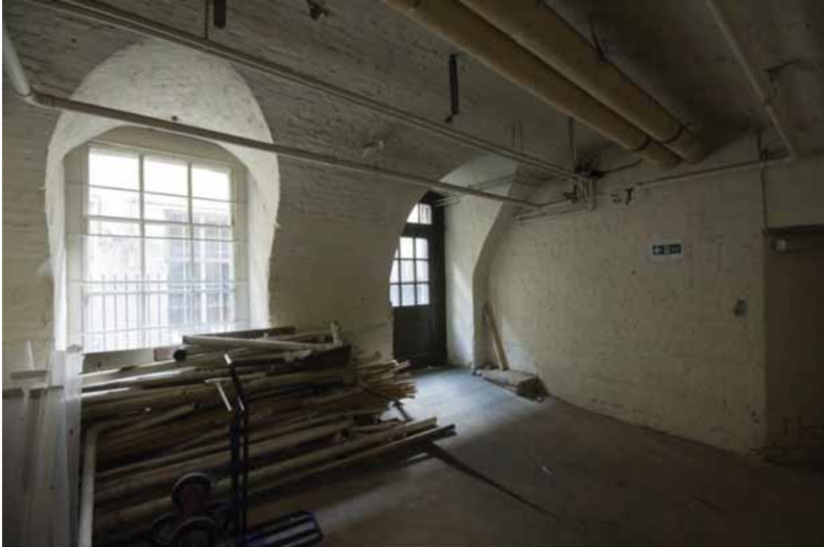
Plate 121: East (left) and south (right) walls in Room B50, looking south-east (DSC_1358 _sitecode EAF10_© PCA Ltd 2010)
