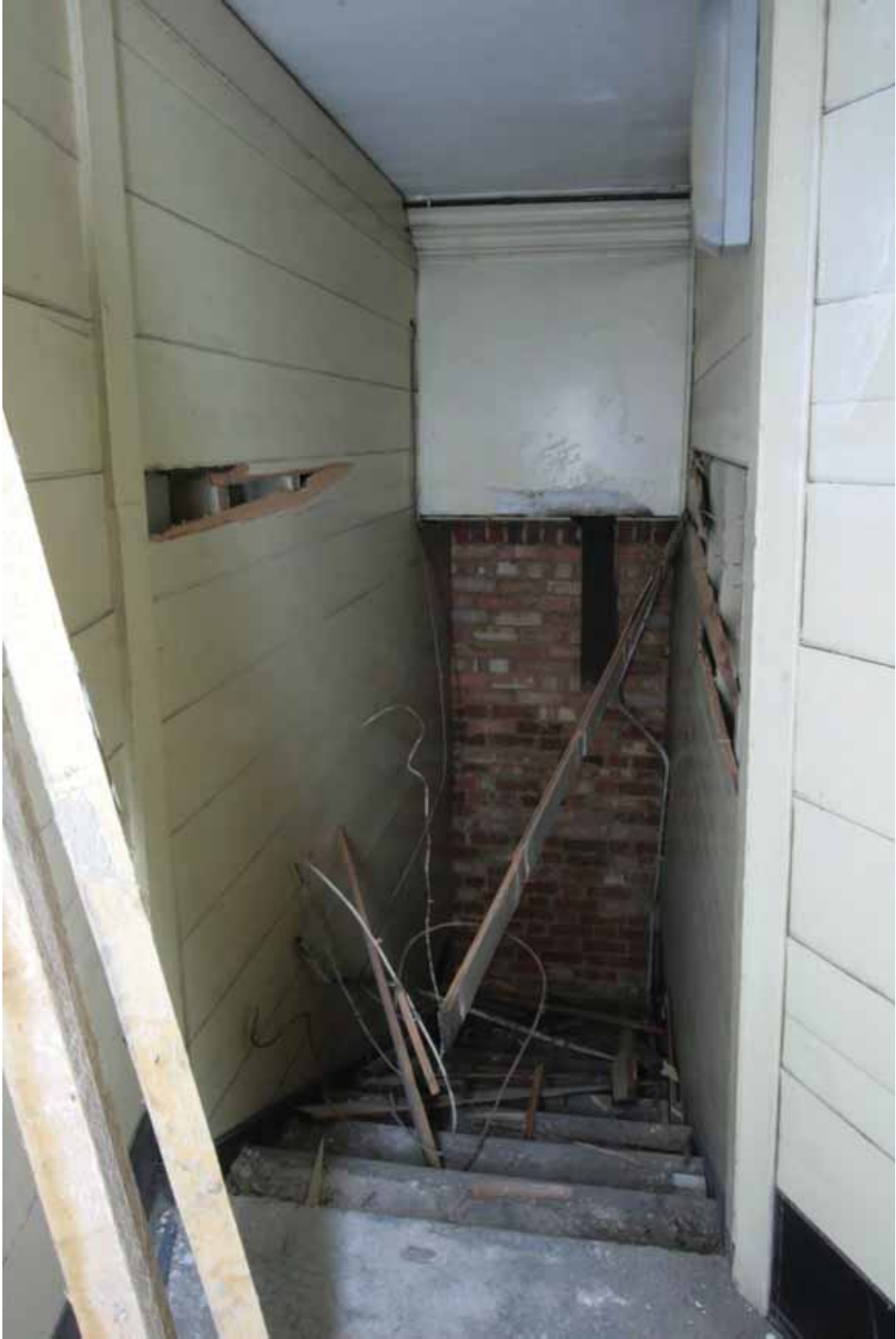
Plate 214c: View down the stairs within Room M18 towards the north wall, looking north (EAF10 237)
