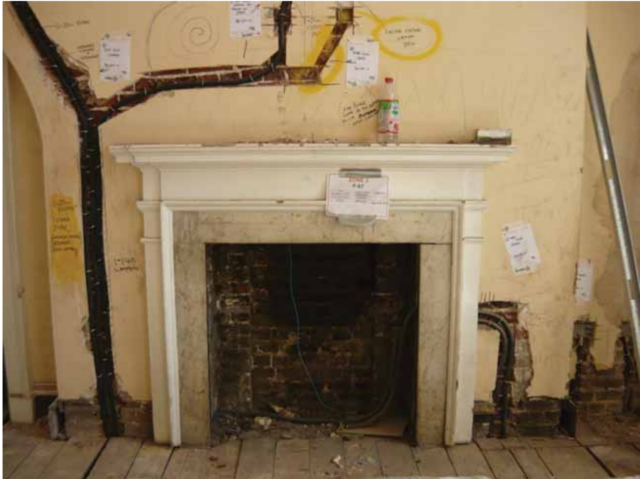
Plate 457b: Fireplace (type 6) in the south wall of Room F67, looking south (EAF10 BHD12 (8))
