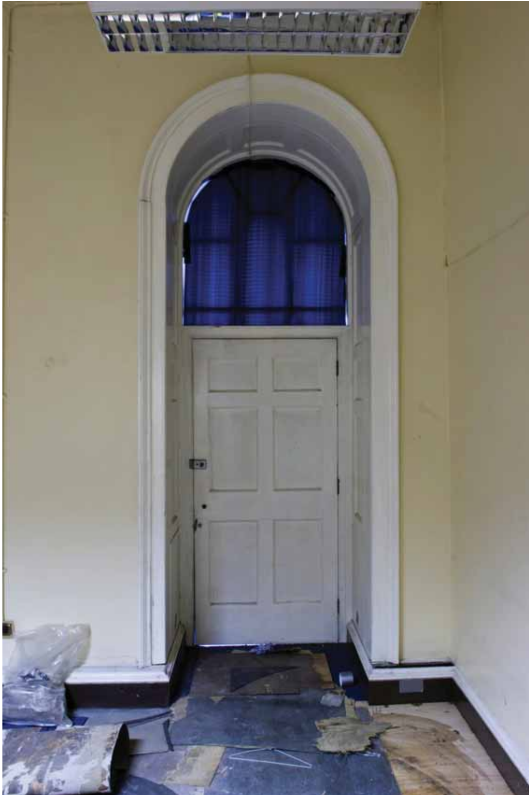
Plate 195: Doorway at the north end of the west wall of Room M14, looking west (DSC_1341 _sitecode EAF10_© PCA Ltd 2010)
