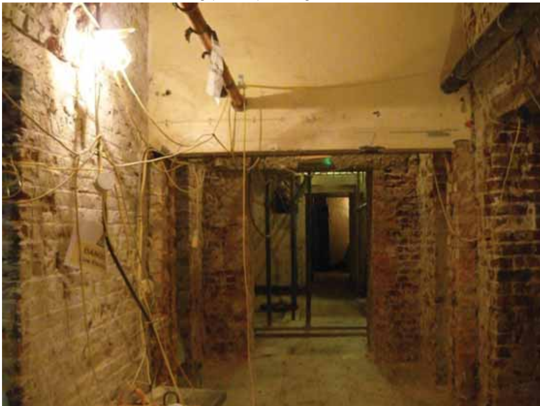
Plate 82: View north from Corridor 1B to Corridor 1A and Stairs 01 (EAF10 BDH6(62))
