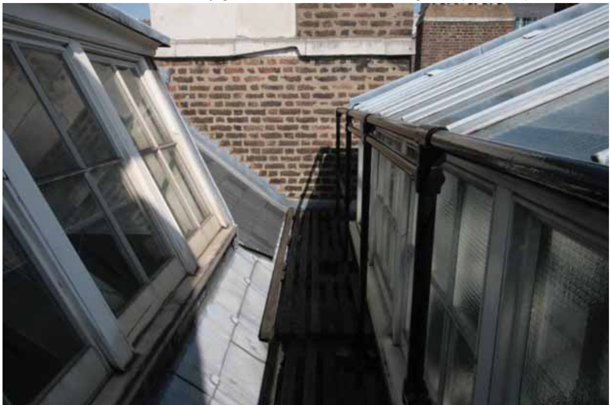
Plate 801: Dormer window over Room T07 (left) and lantern skylight over the Corridor 02T (right), looking north (EAF10 23)
