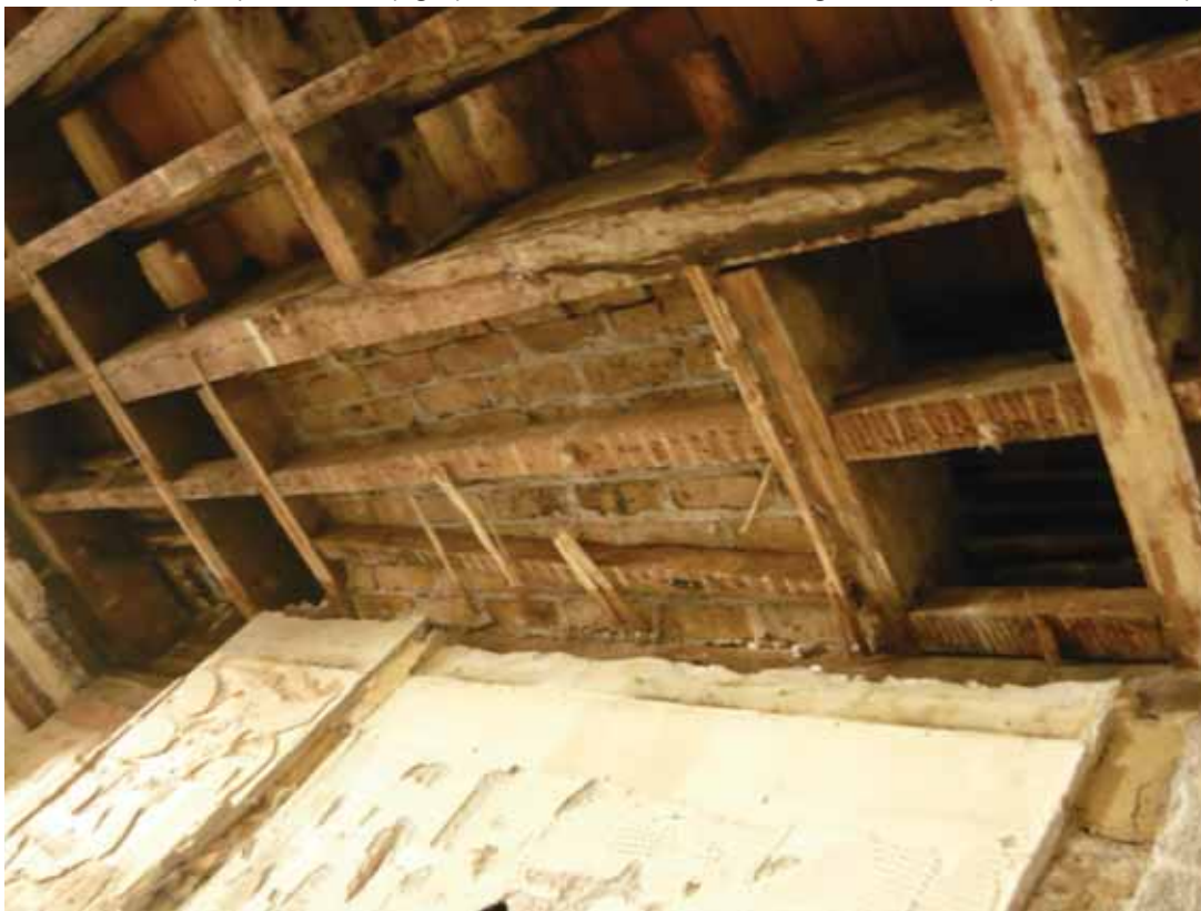
Plate 638: Brickwork under the hearthstone adjacent to the top of the south wall in Room S20, looking south-east (EAF10 BHD8 (47))
