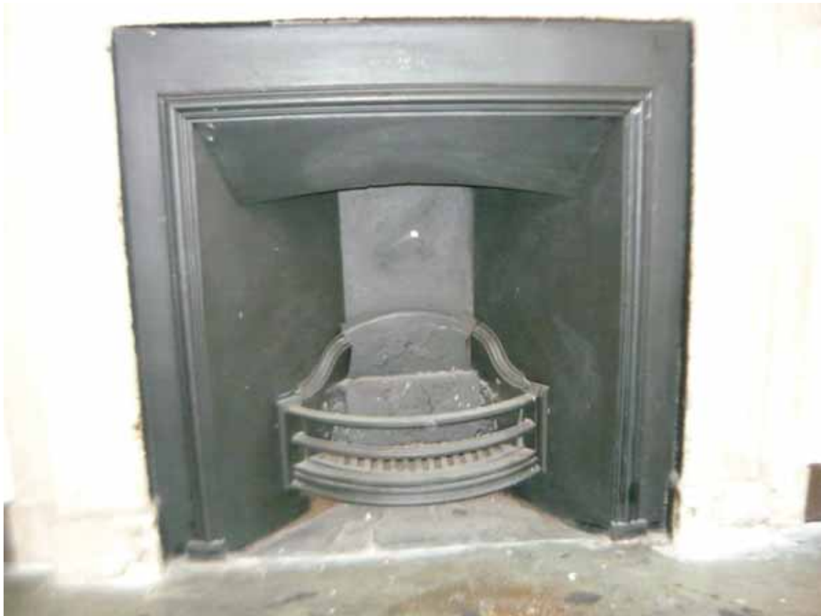
Plate 420: Close up of the fireplace in the north wall of Room G18, looking south-west (EAF10 B100 0876)
