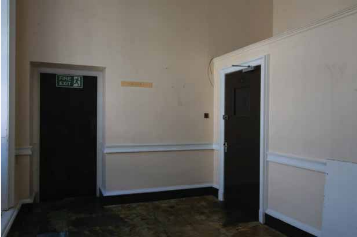
Plate 544: South (left and centre) and west partition (right) walls in Room F27, looking south-west (EAF10 154)
