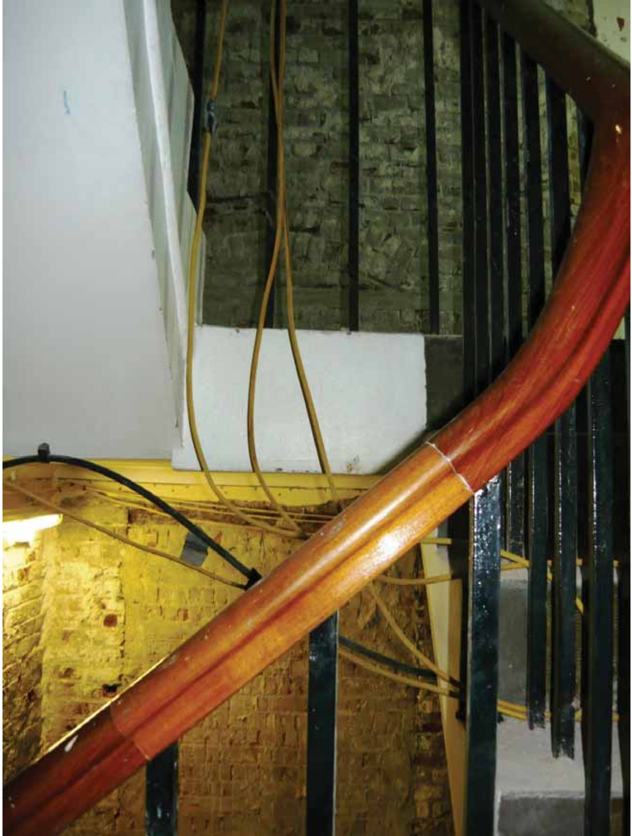
Plate 248: North end of the east wall in Corridor 06LG looking east (EAF10 BHD7 (9))
