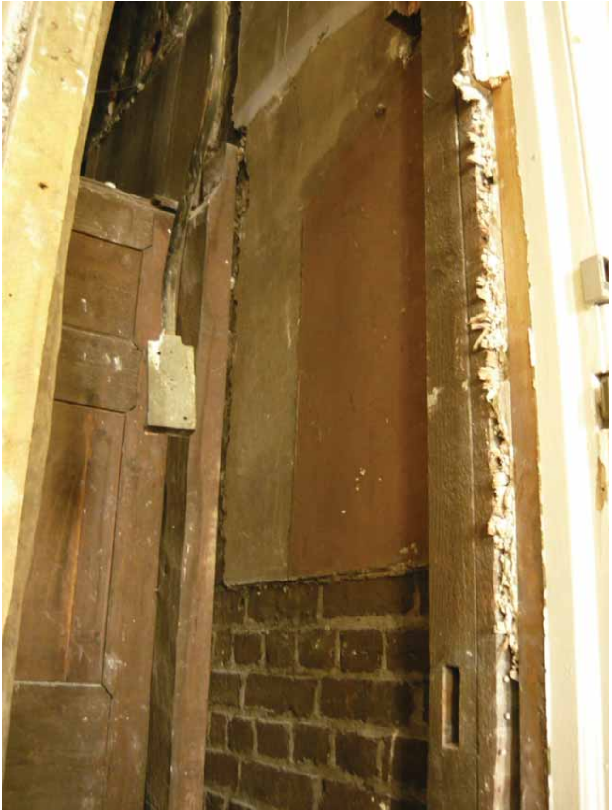
Plate 524: Void at the north end of the partition wall in Room F16, looking north-west (EAF10 BHD8 (26))
