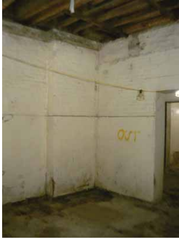
Plate 49: East (left) and south (right) walls in Room B48A, looking south-east (EAF10 BHD5 (11))
