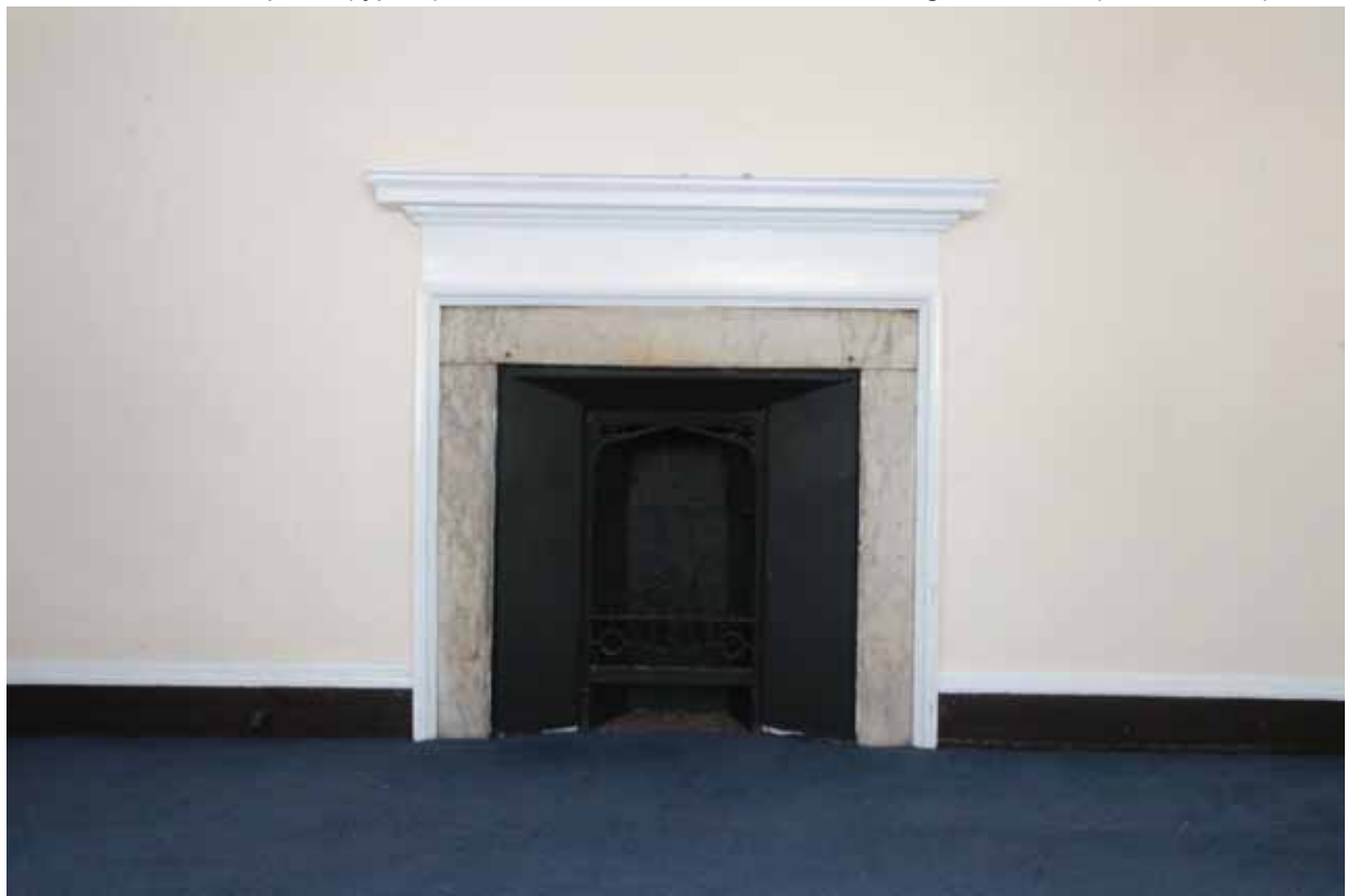
Plate 587: Fireplace (type 2) in the south wall of Room S15, looking south (EAF10 0101)
