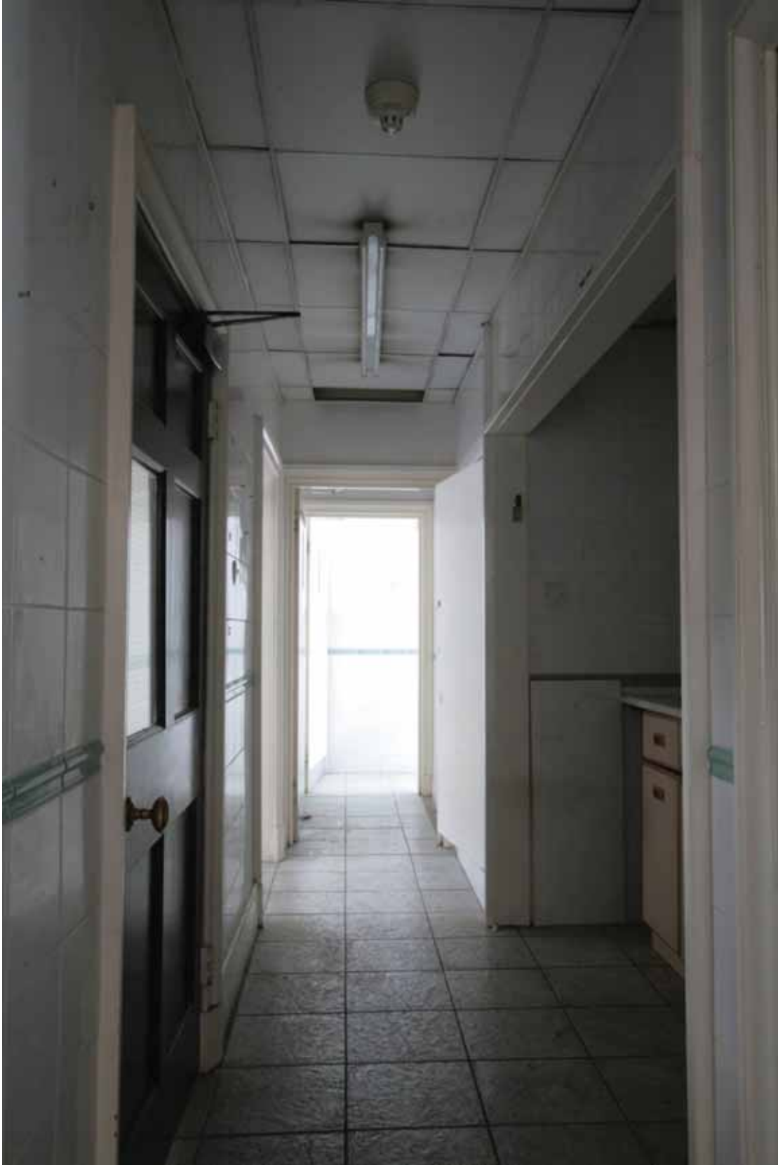
Plate 631: West (left) and east partition (right) walls in Room S20, looking north (EAF10 0122)
