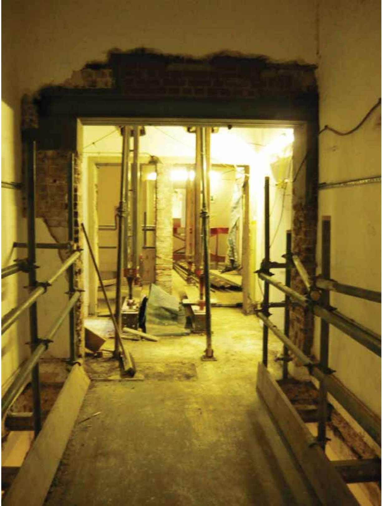
Plate 402: Widening of the north doorway in Corridor 09G during the current works, looking north (EAF10 BHD8 (129))
