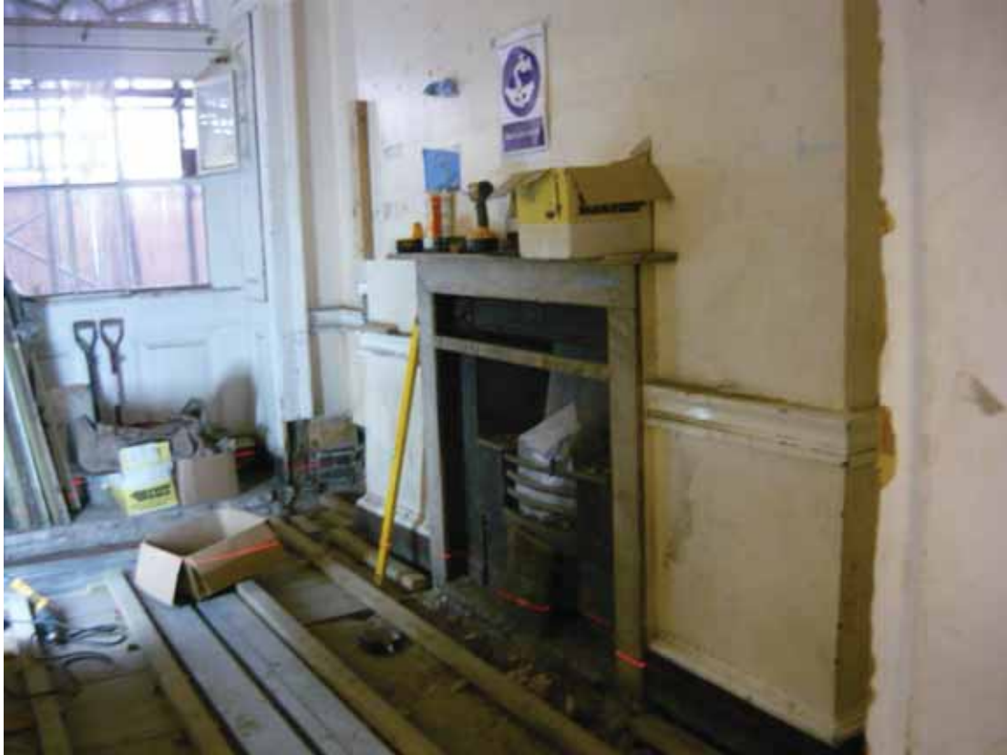
Plate 436: East (left) and south (right) walls in Room G23, looking south-east (EAF10 BHD13 (7))
