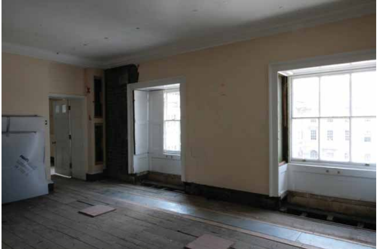
Plate 558: South (left) and west (right) walls in Room S95, looking south-west (EAF10 232)
