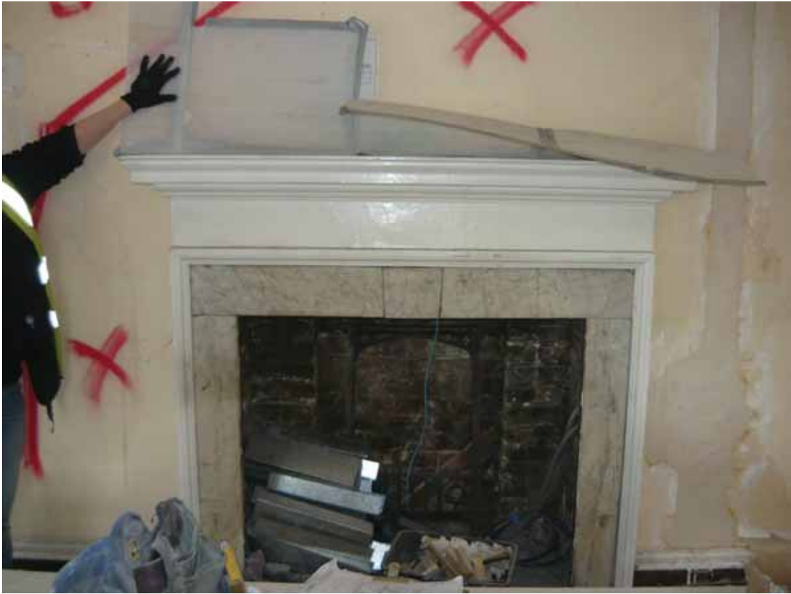
Plate 581: Fireplace (type 1) in the east wall of Room S10, looking east (EAF10 BHD12 (1))
