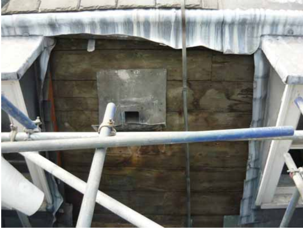
Plate 808: Slates stripped from the east side of the east wall between two sash windows (left for Room T15 and right for Room T16, looking east (EAF10 BHD9 (11))
