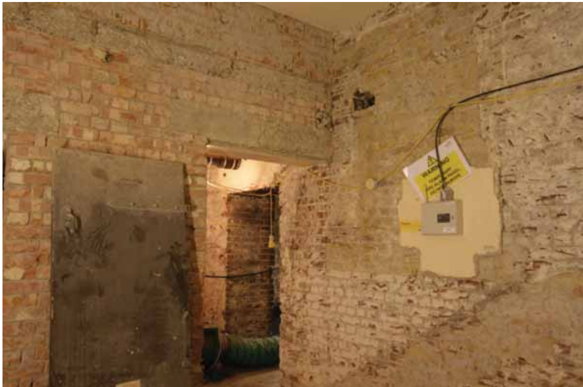
Plate 88: North (left) and east (right) walls of Corridor 2, looking north-east (EAF10 A100 043)
