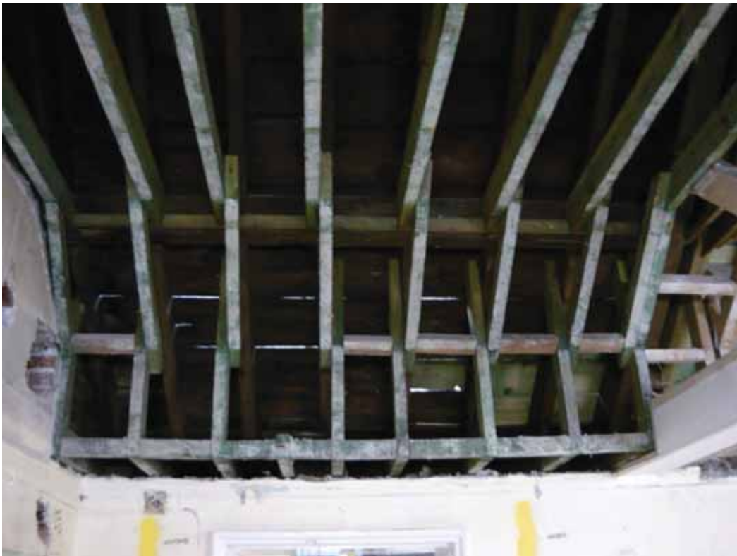
Plate 735: Roof structure above the south end of the west wall of Room T117, looking west (EAF10 BHD10 (38))
