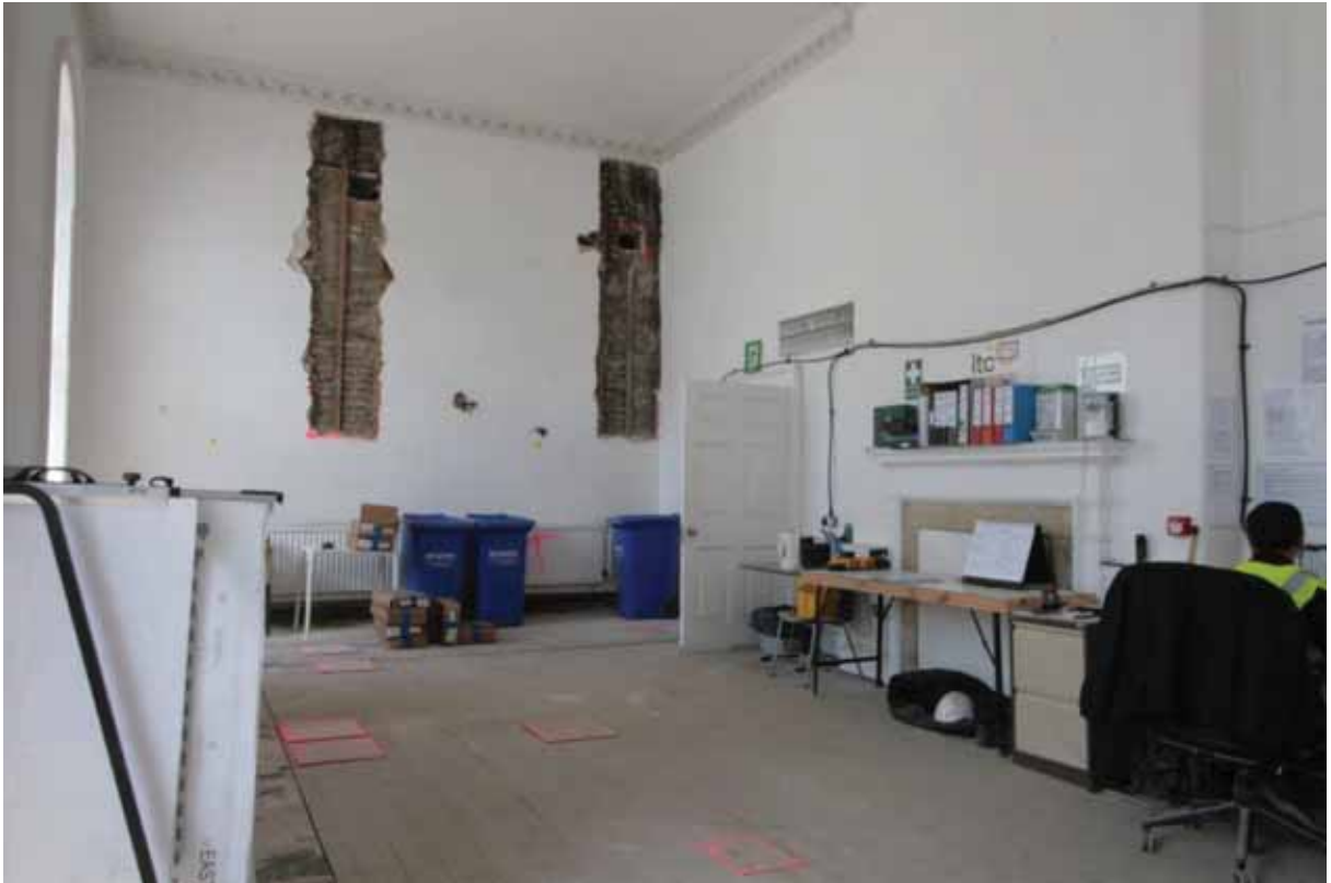
Plate 374: North (left) and east (right) walls in Room G09, looking north-east (EAF10 266)
