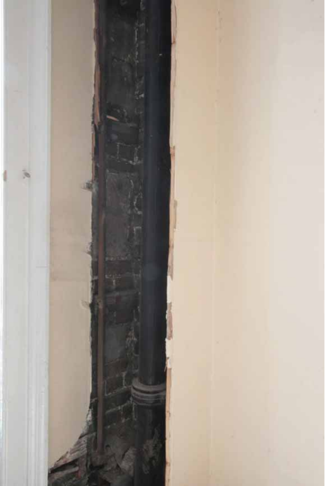
Plate 210: Cast iron pipe in the north-west corner of Room M16, looking north-west (EAF10 309)
