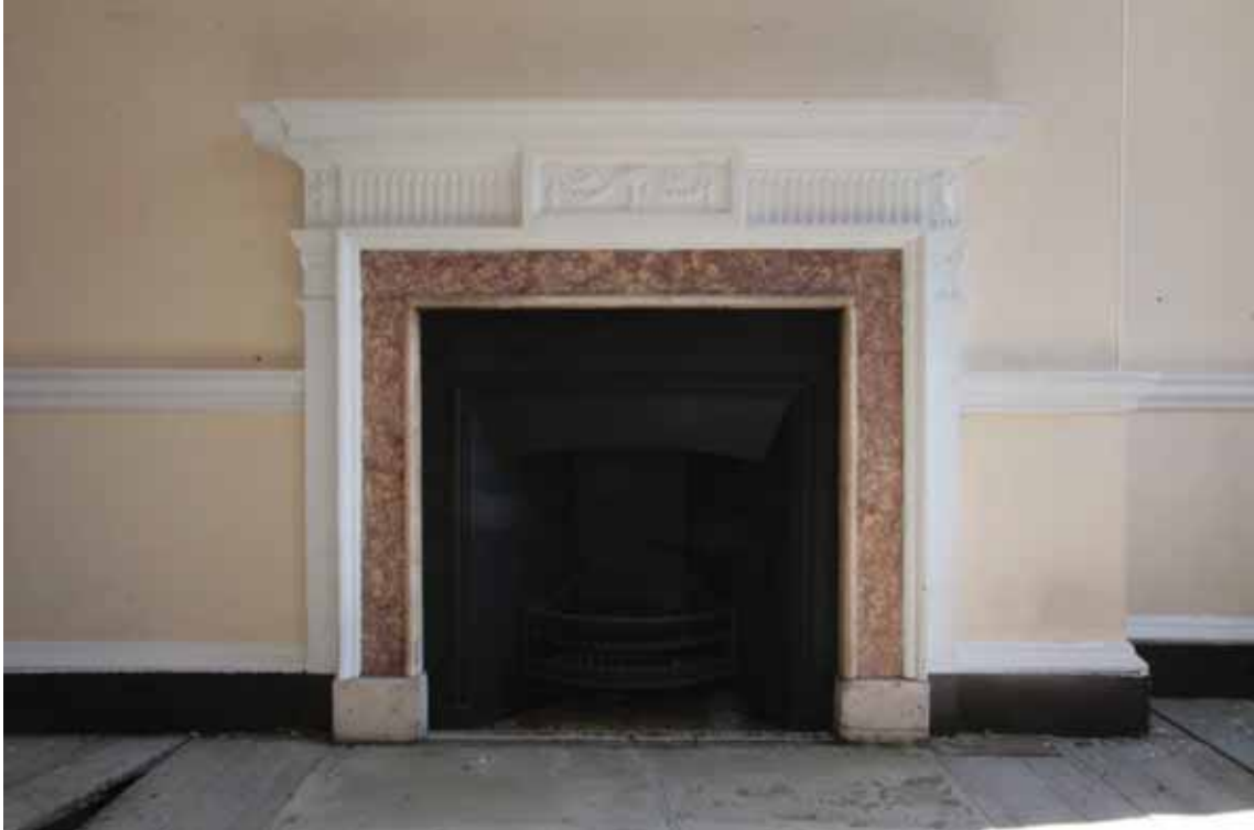
Plate 464a: Fireplace (type 8) in the south wall of Room F02, looking south (EAF10 181)
