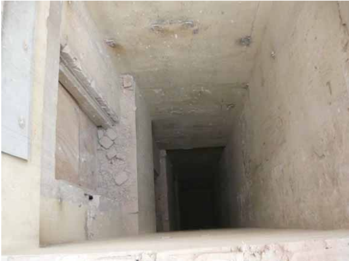
Plate 715: North (left), east (centre) and south (right) walls of the lift, looking east and down from the east side of Corridor 04T to the second floor and below (EAF10 BHD (51))
