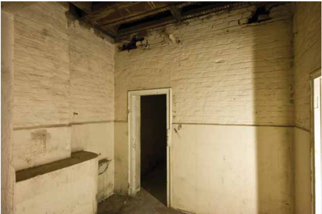
Plate 44: East (left) and south (right) walls of Room B48B, looking south-east (DSC_1412 _sitecode EAF10_© PCA Ltd 2010)
