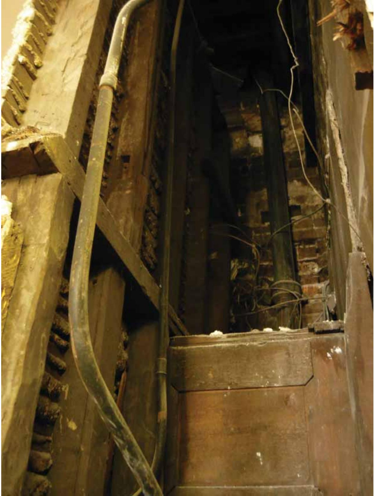
Plate 521: Void at the north end of the partition wall in Room F16, looking up and west (EAF10 BHD8 (34))
