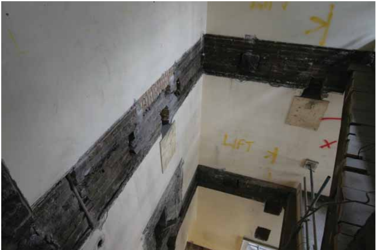
Plate 705: South (left) and west (right) walls in Room T14, looking south-west (EAF10 A100 002)
