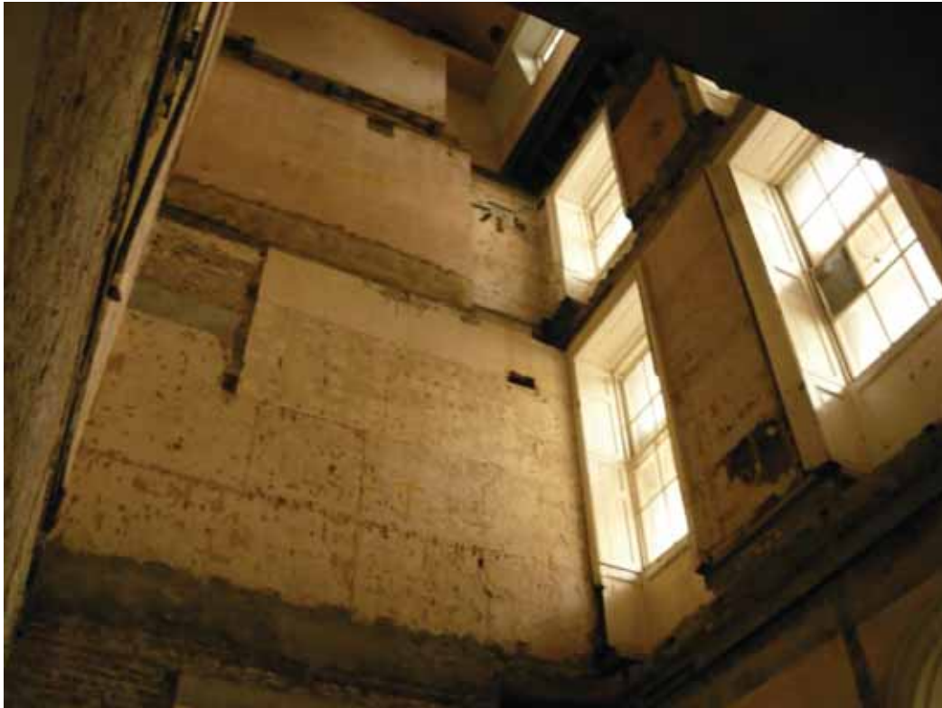
Plate 535: North (left) and east (right) walls in Room F20, looking up and north-east (EAF10 BHD8 (86))
