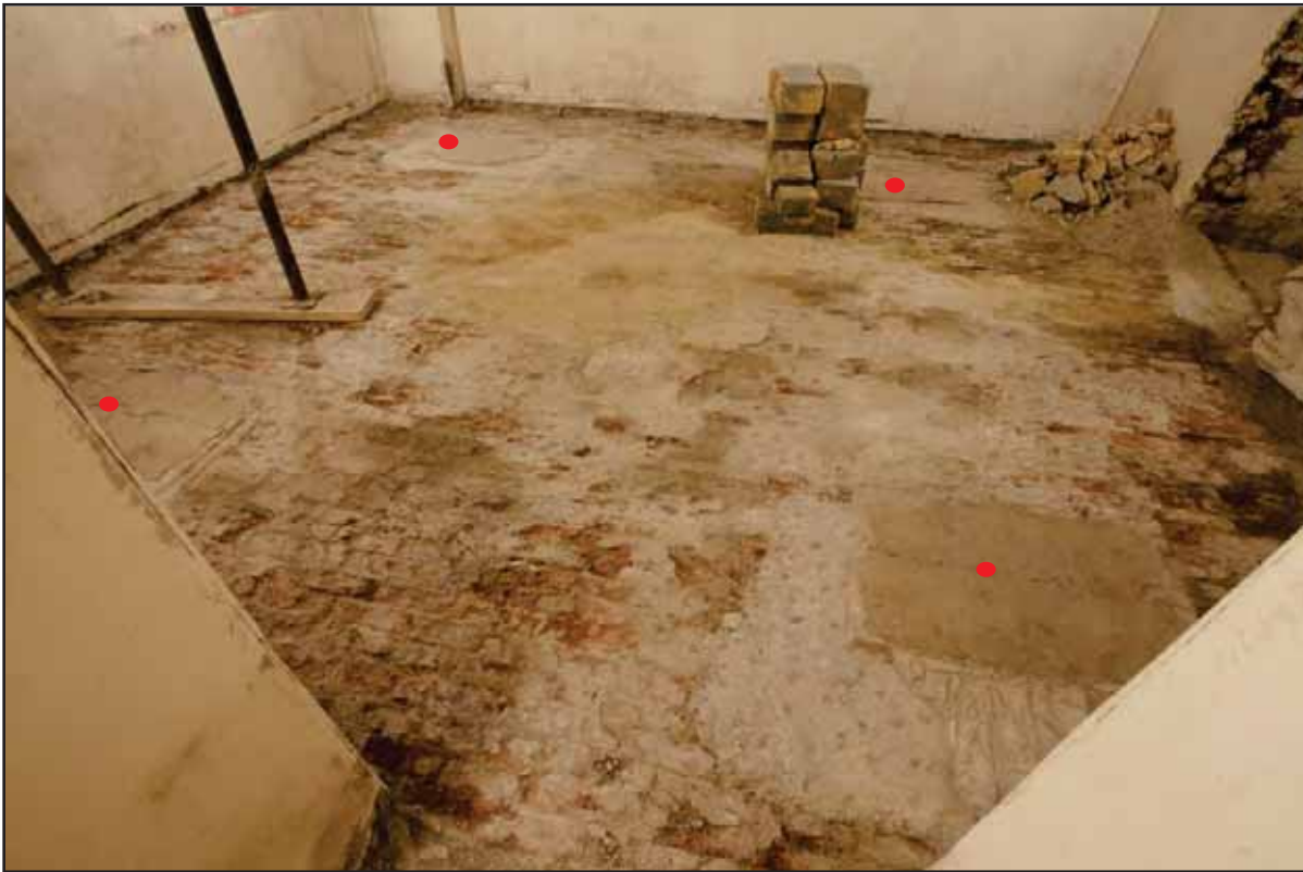
Plate 59: Original brick floor in room B48A with World War 2 shoring foundations (marked with red dots), looking north-west (IMG_0003-2)
