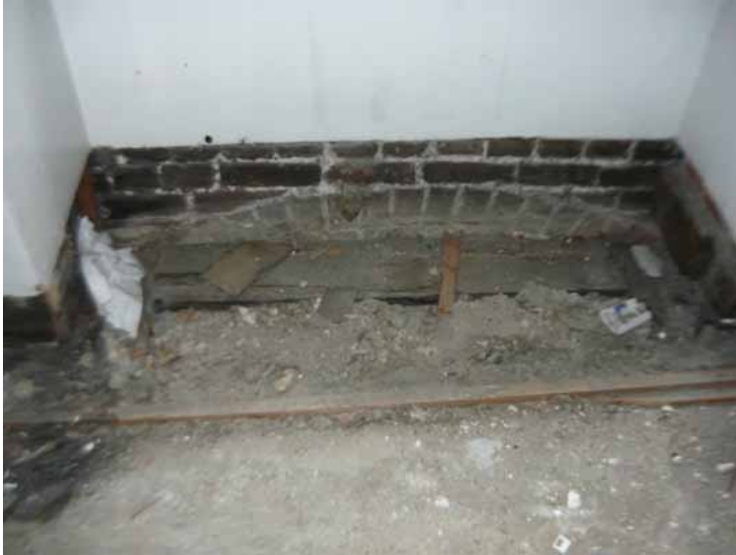
Plate 269: Brick arch below the south window in the east wall of Room M20, looking east (EAF10 BHD3 (67))
