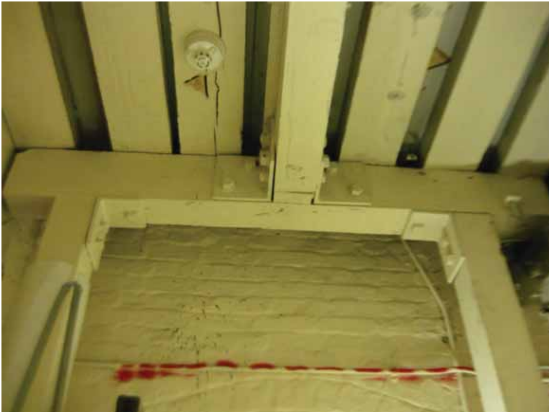
Plate 20a: Second world War timber shoring above the door in Room B45, looking north (EAF10 BHD1 (128))
