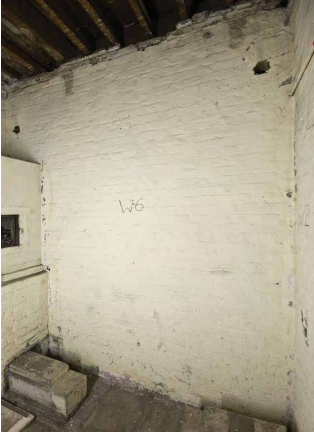
Plate 23: West wall of Room B45, looking west (DSC_1372 _sitecode EAF10_© PCA Ltd 2010)
