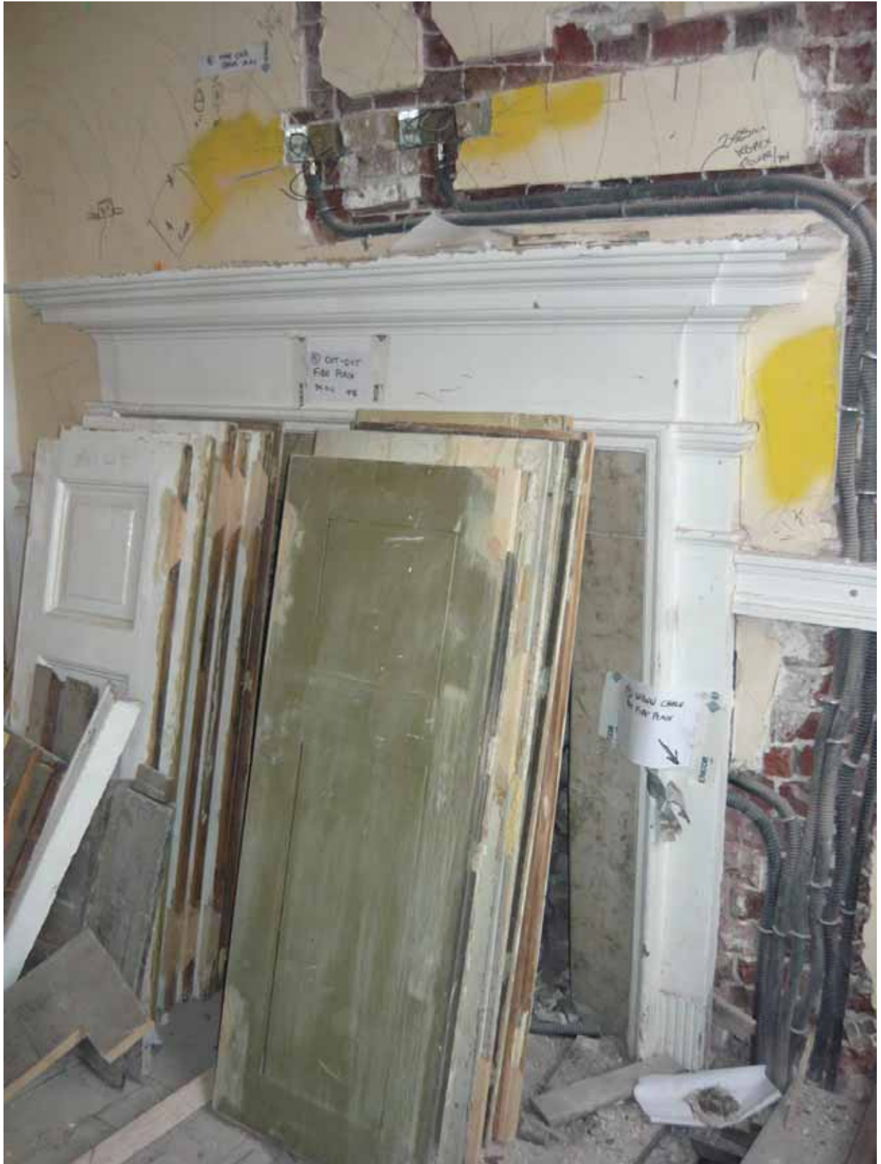
Plate 543b: Fireplace (type 6) in the south wall of Room F26, looking south-east (EAF10 BHD12 (14))
