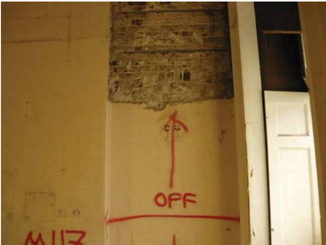
Plate 334: East end of the north wall in Room M117, looking north (EAF10 BHD6 (101))
