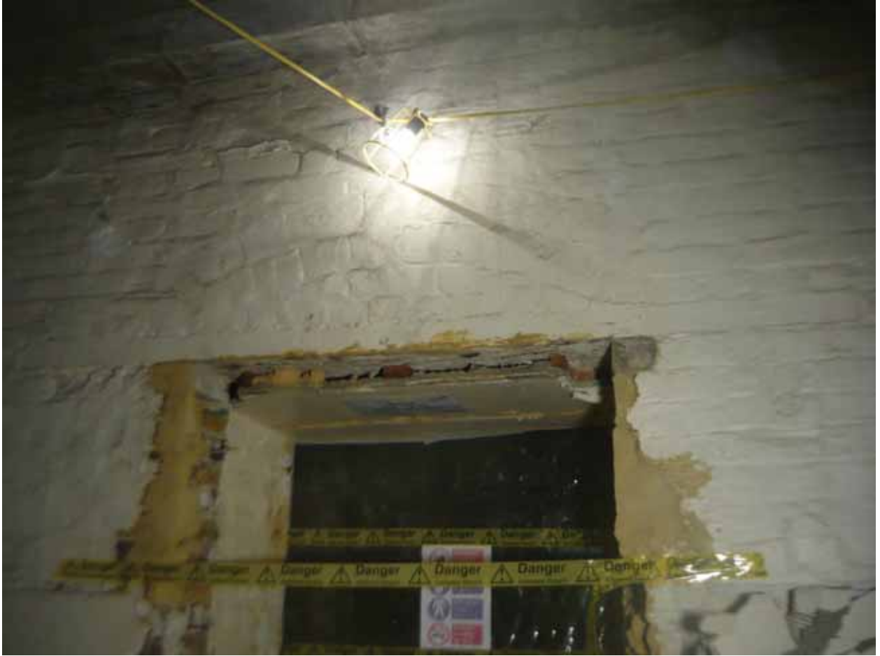
Plate 62: Doorway at the north end of the east wall in Room B48A, looking east (EAF10 BHD5 (18))
