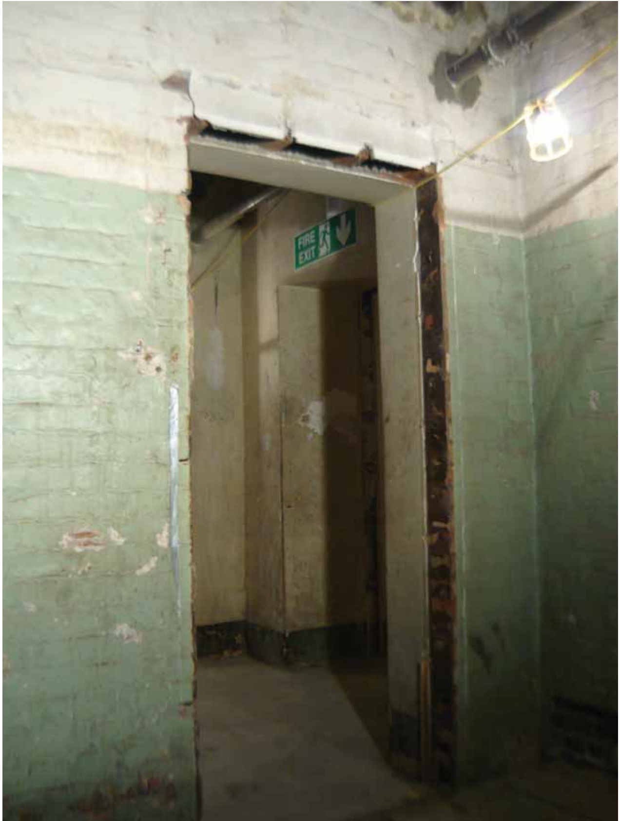
Plate 156: Doorway in the south wall of Room B54A, looking south-west (EAF10 BHD5 (181))
