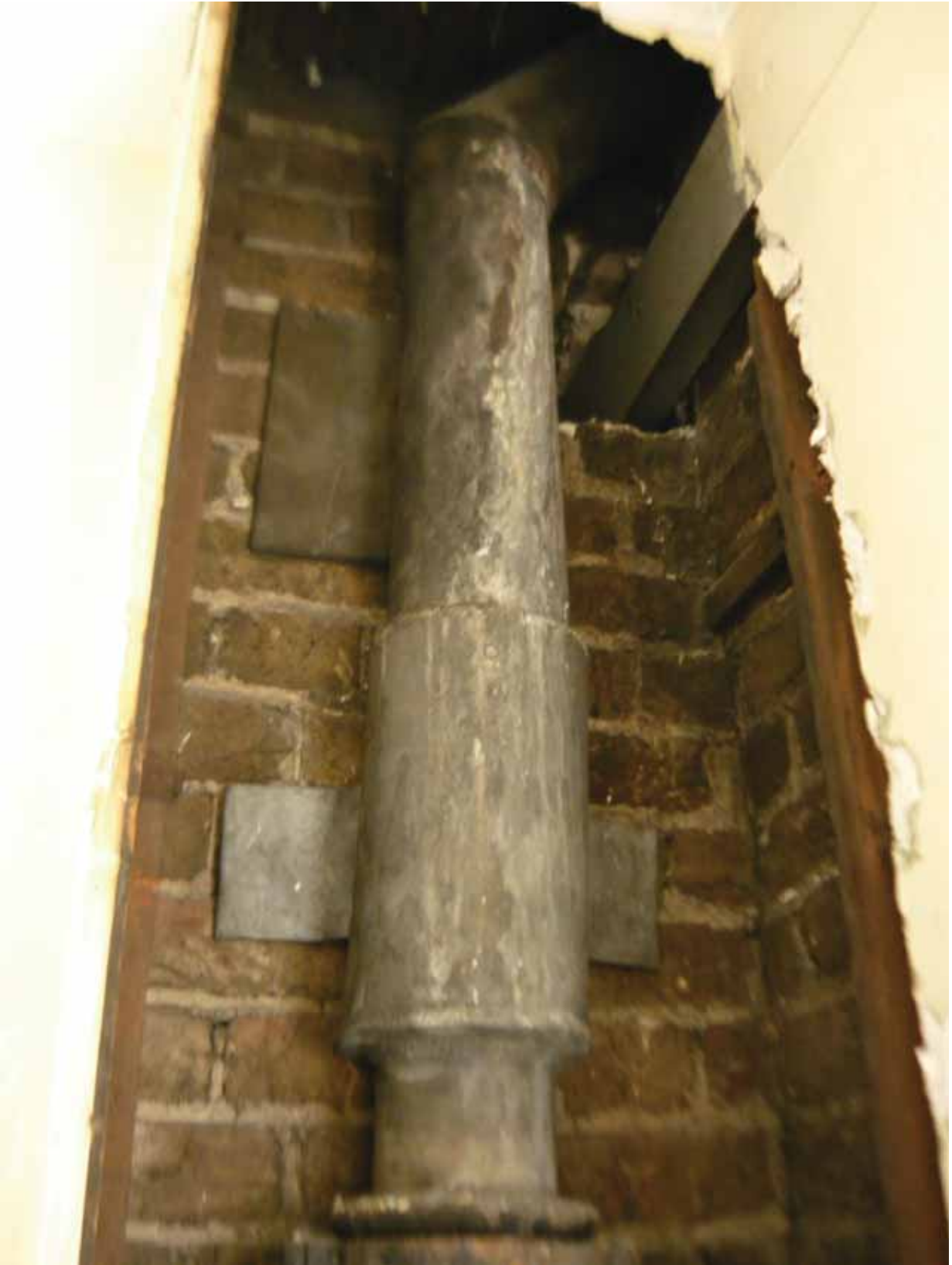
Plate 574: Upper part of boxed in pipe in the south-west corner of Room S08, looking south (EAF10 BHD2 (65))
