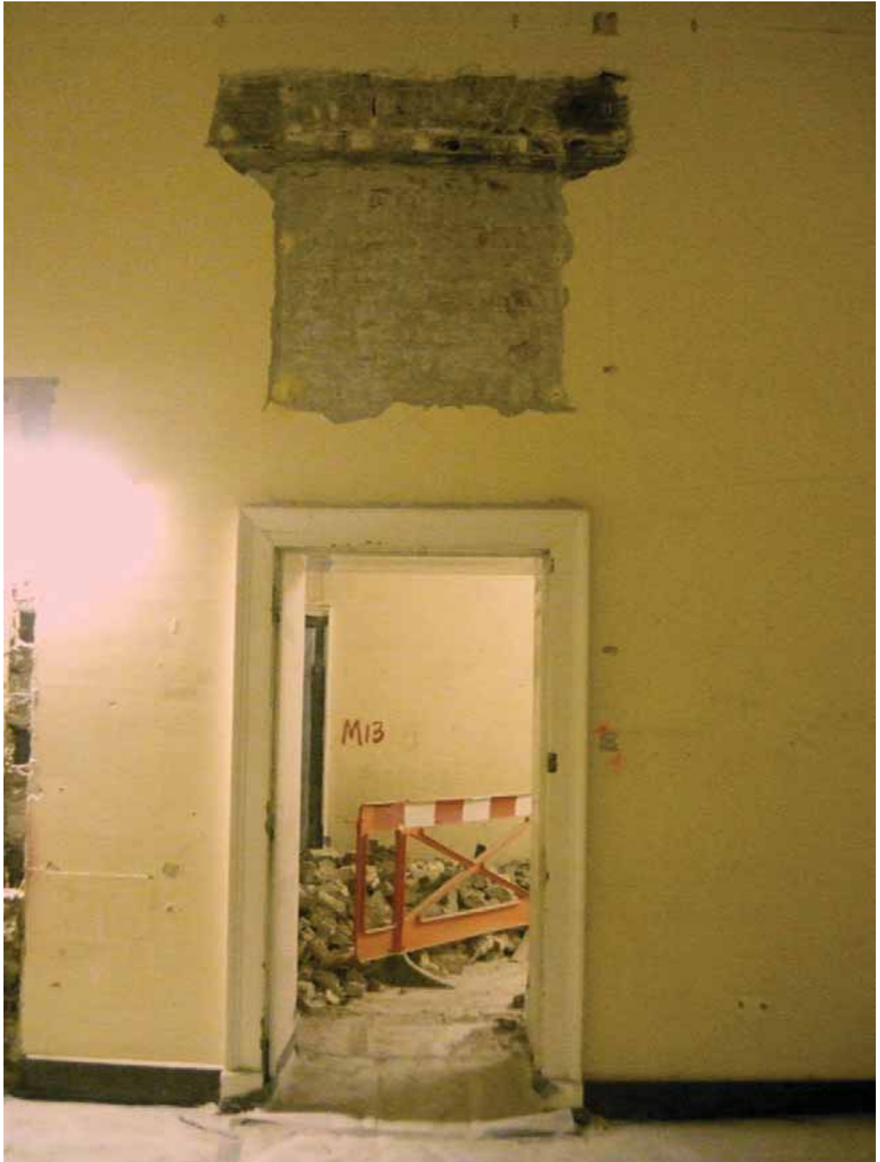
Plate 280: Doorway in the west wall of Room M23, looking west (EAF10 BHD6 (72))
