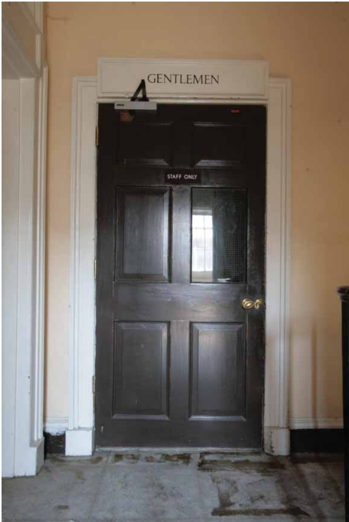
Plate 500: Doorway at the north end of the east wall in Corridor 05F looking east (EAF10 184)
