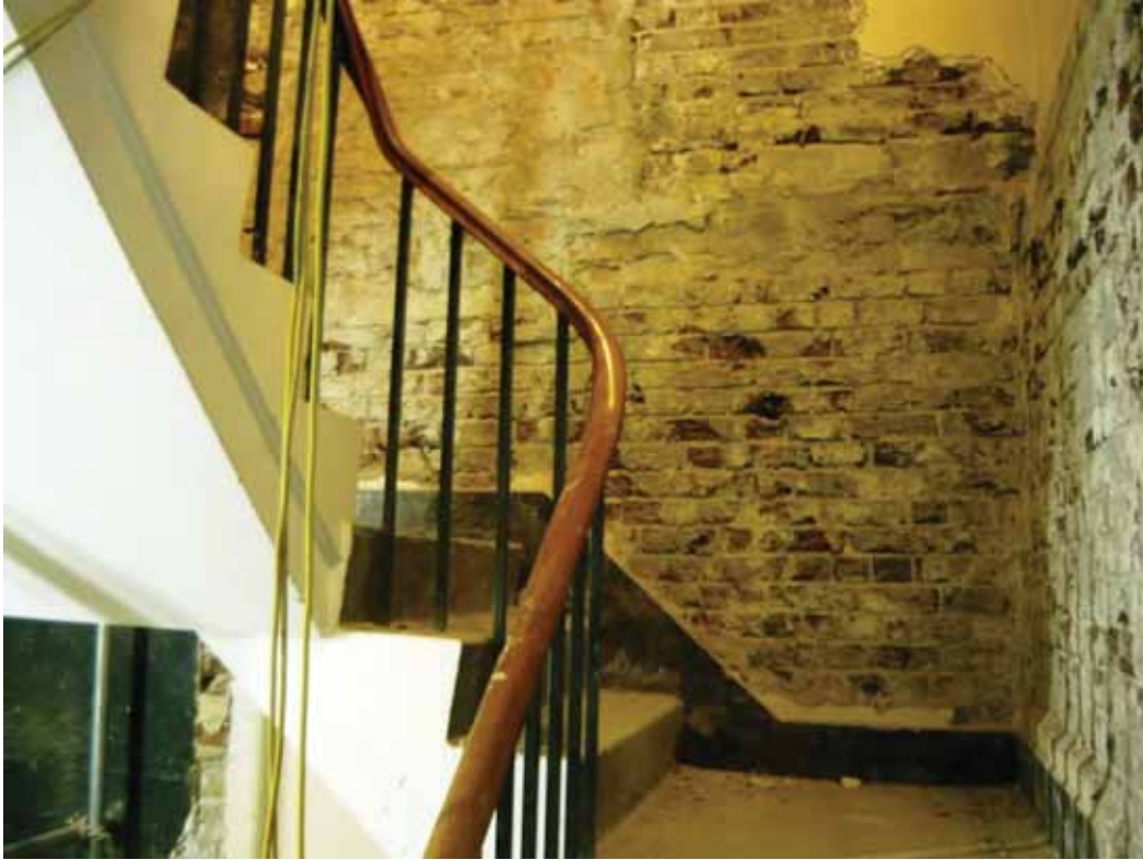
Plate 251: West (left and centre) and north (right) walls (upper level) in Corridor 06LG looking west (EAF10 BHD7 (12))
