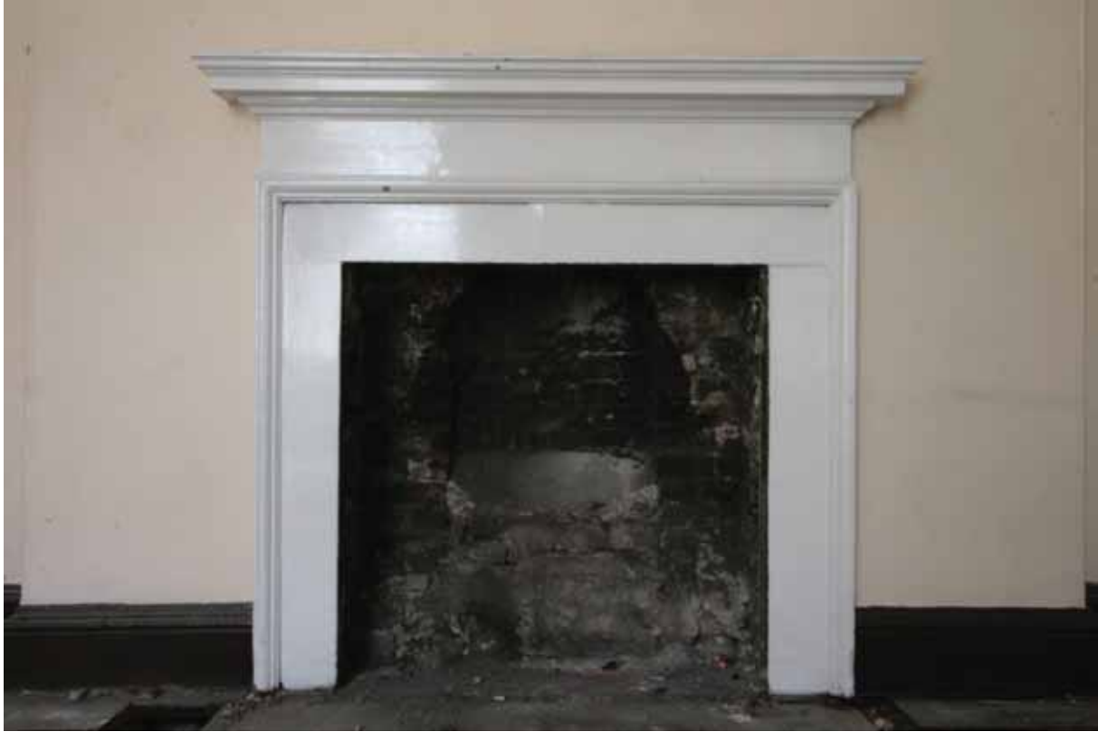
Plate 177: North fireplace (type 2) in the east wall of Room M08, looking east (EAF10 303)
