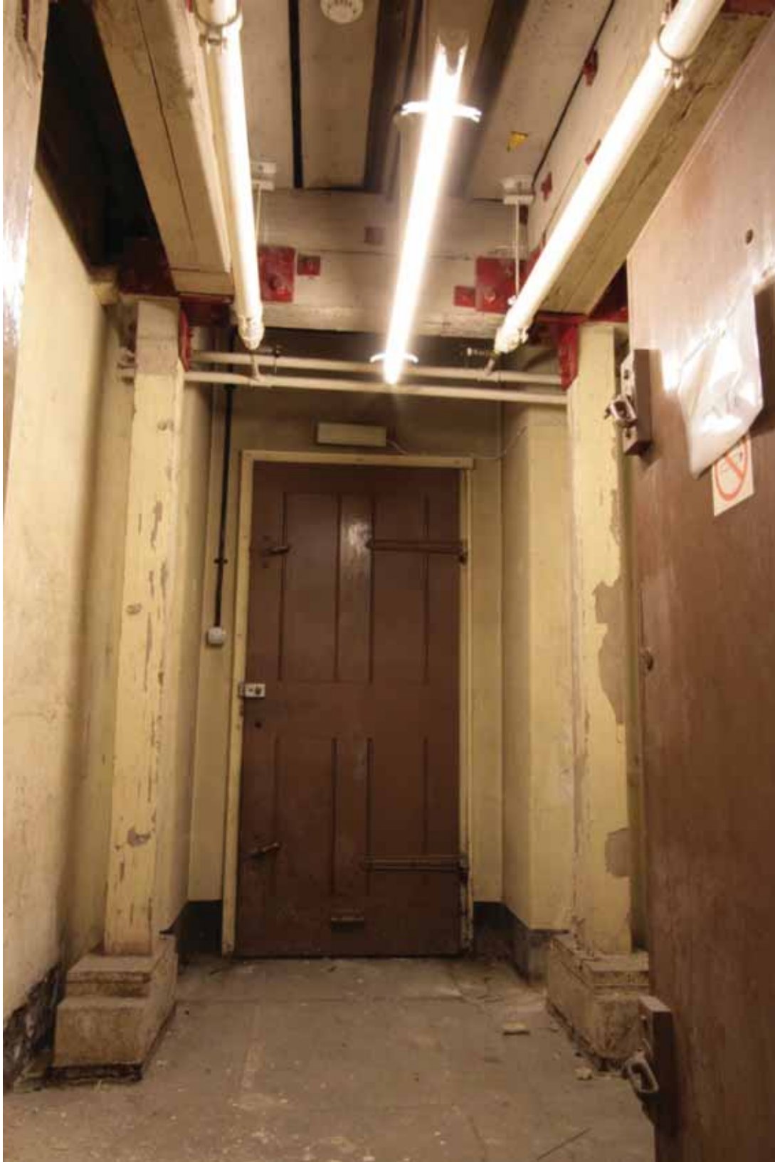
Plate 165a: Doorway in the east wall of Room B54A, looking east (DSC_1491 _sitecode EAF10_© PCA Ltd 2010)
