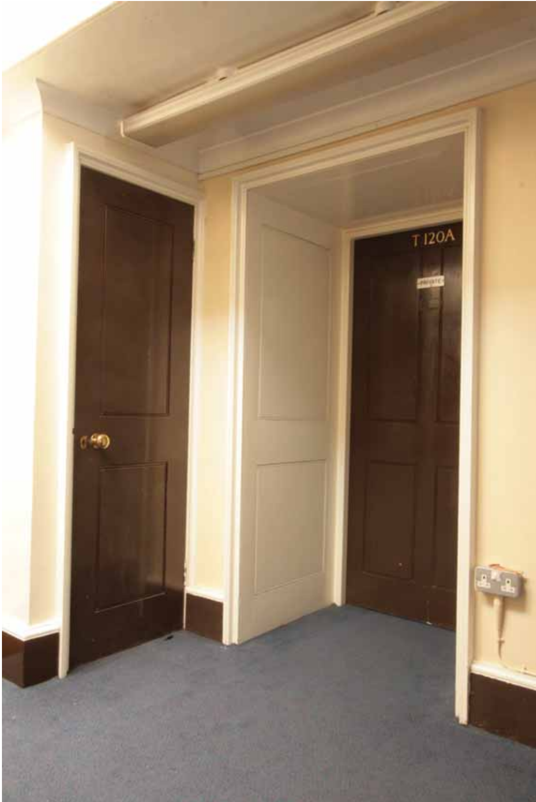
Plate 727: Doorway (left) in south partition wall and doorway (right) in west wall of Corridor 10T, looking south-west (EAF10 56)
