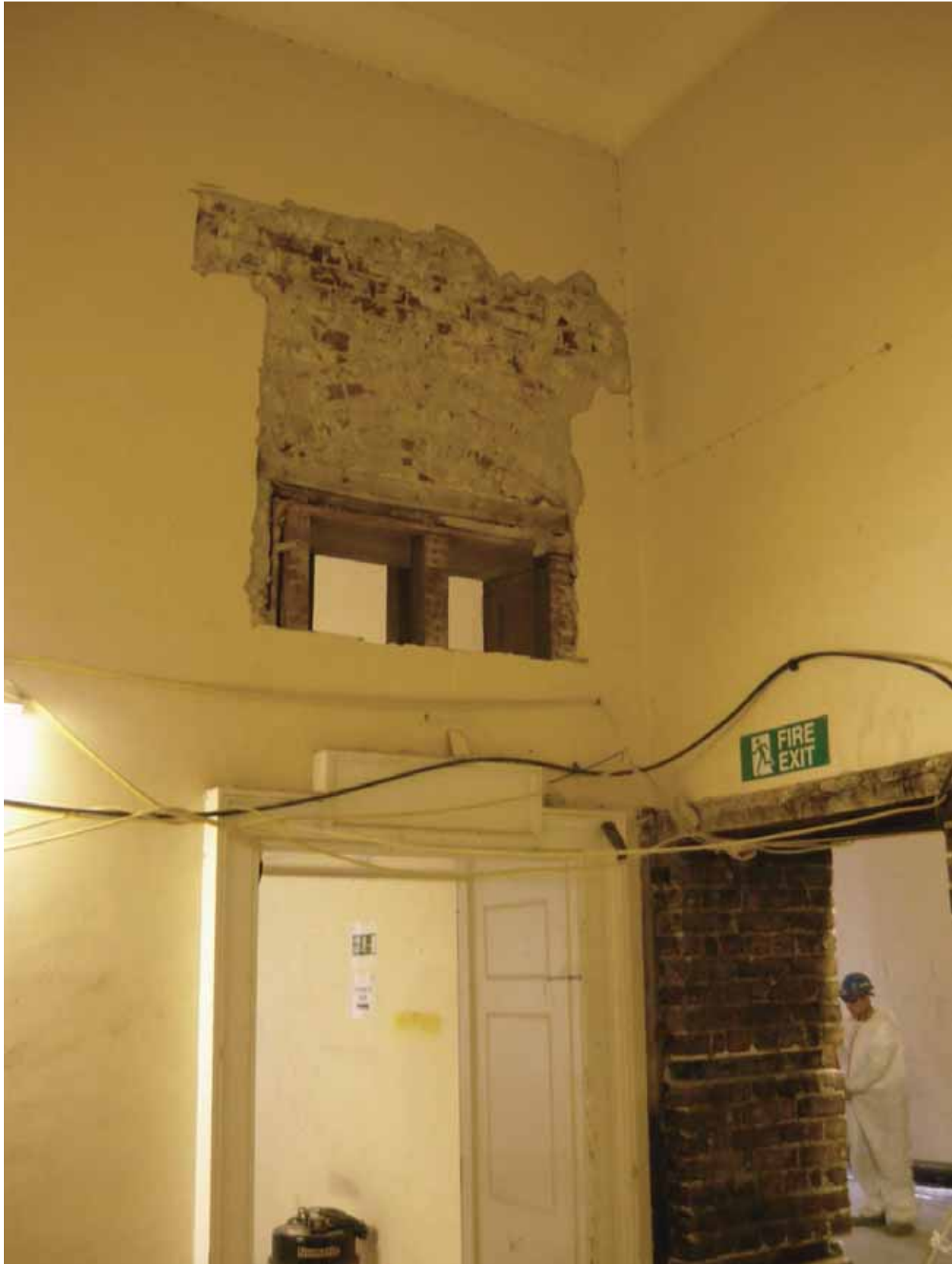
Plate 239d: East (left) and south (right) walls of Corridor 05LG looking south-east (EAF10 BHD6 (23))
