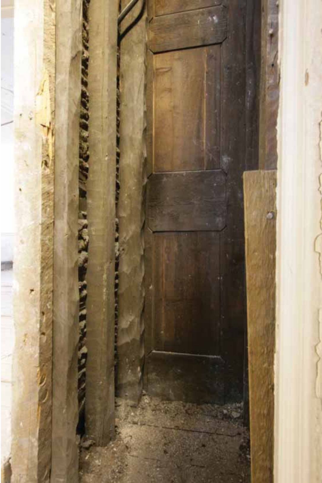
Plate 520: Void at the north end of the partition wall in Room F16, looking west (EAF10 A100 021)
