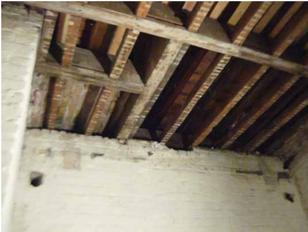
Plate 42: Primary and secondary floor joists visible following the removal of the lath and plaster ceiling in Room B47B, looking west (EAF10 BHD5 (105))
