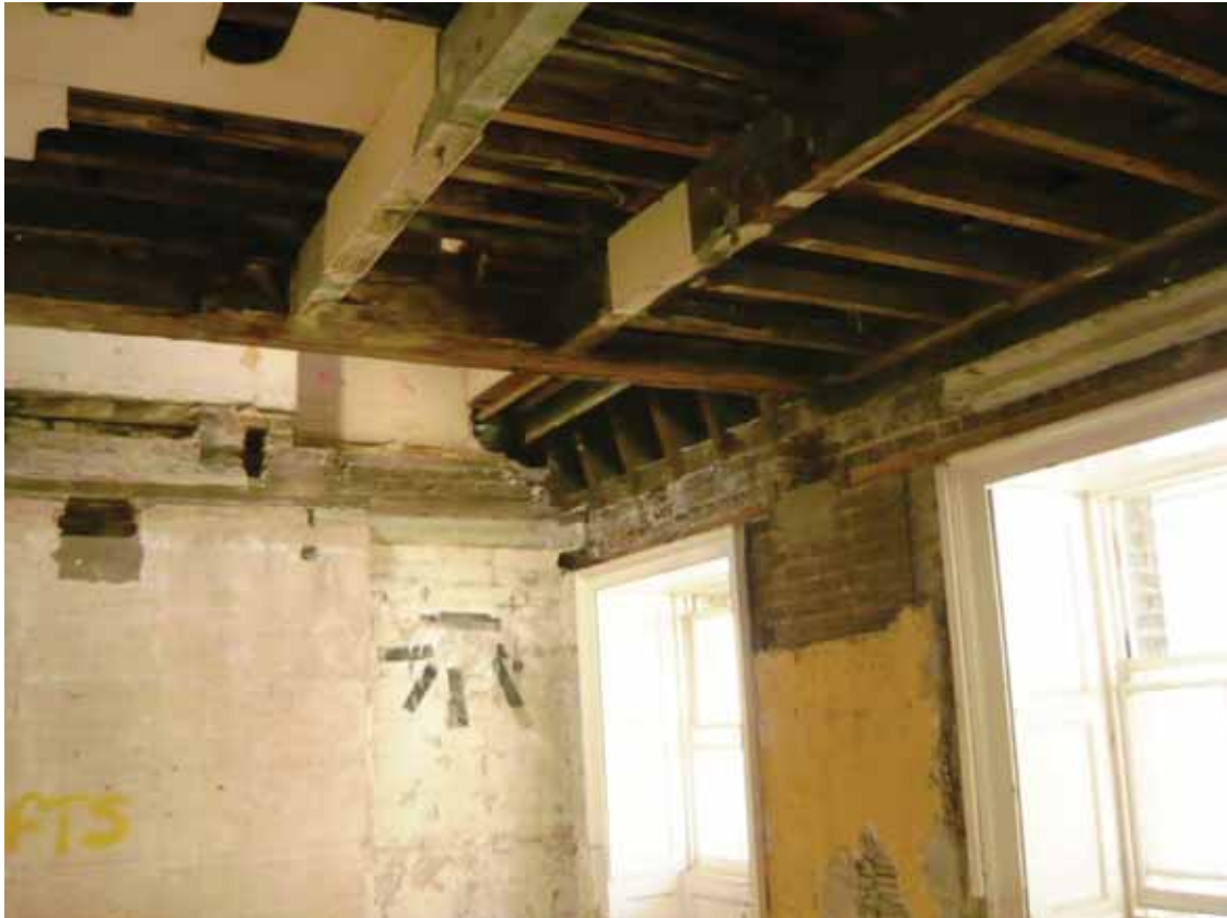
Plate 635: North (left) and east (right) walls in Room S20, looking north-east (EAF10 BHD8 (46))
