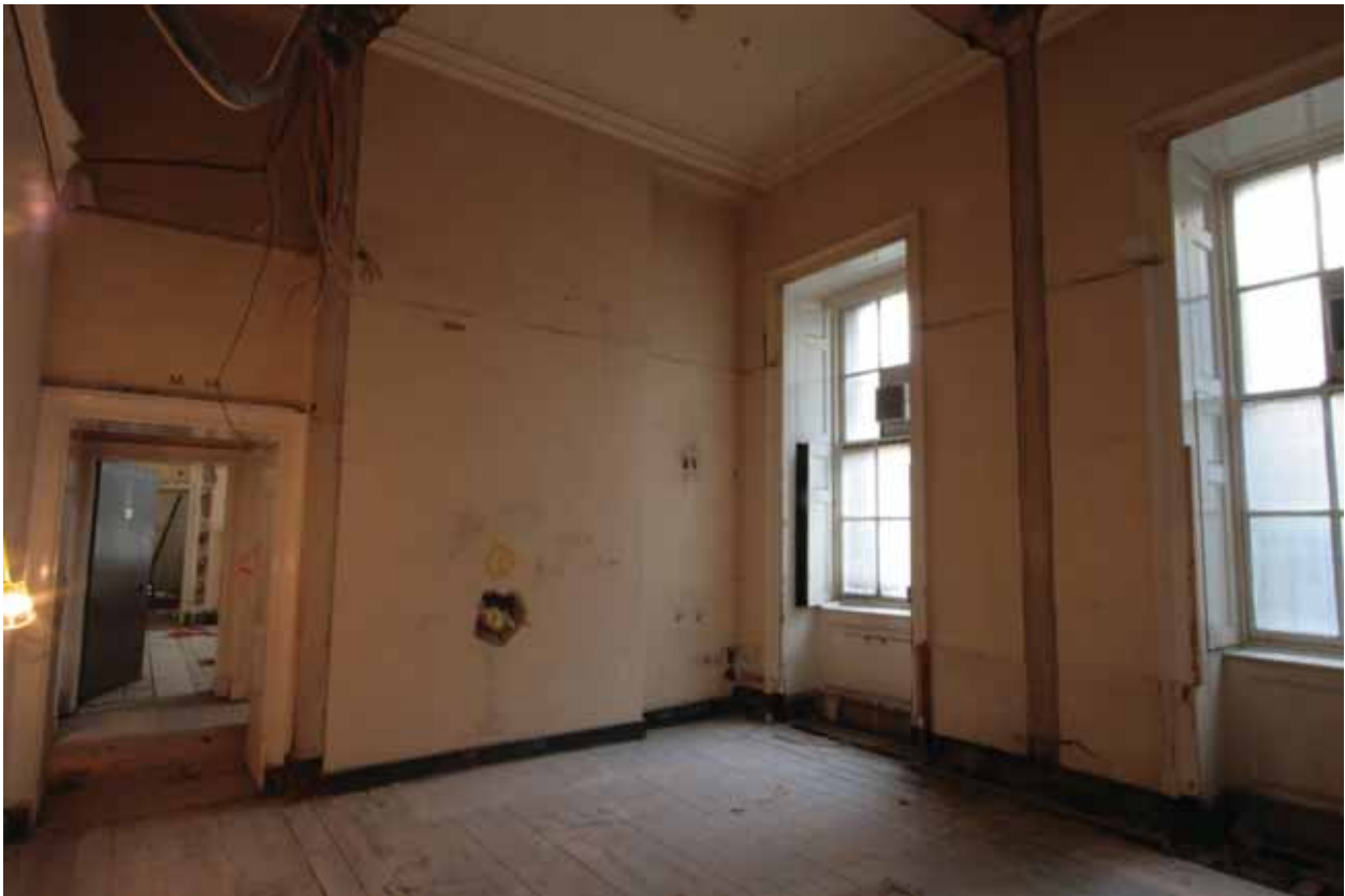
Plate 331: North (left) and east (right) walls in Room M117, looking north-east (EAF10 302)
