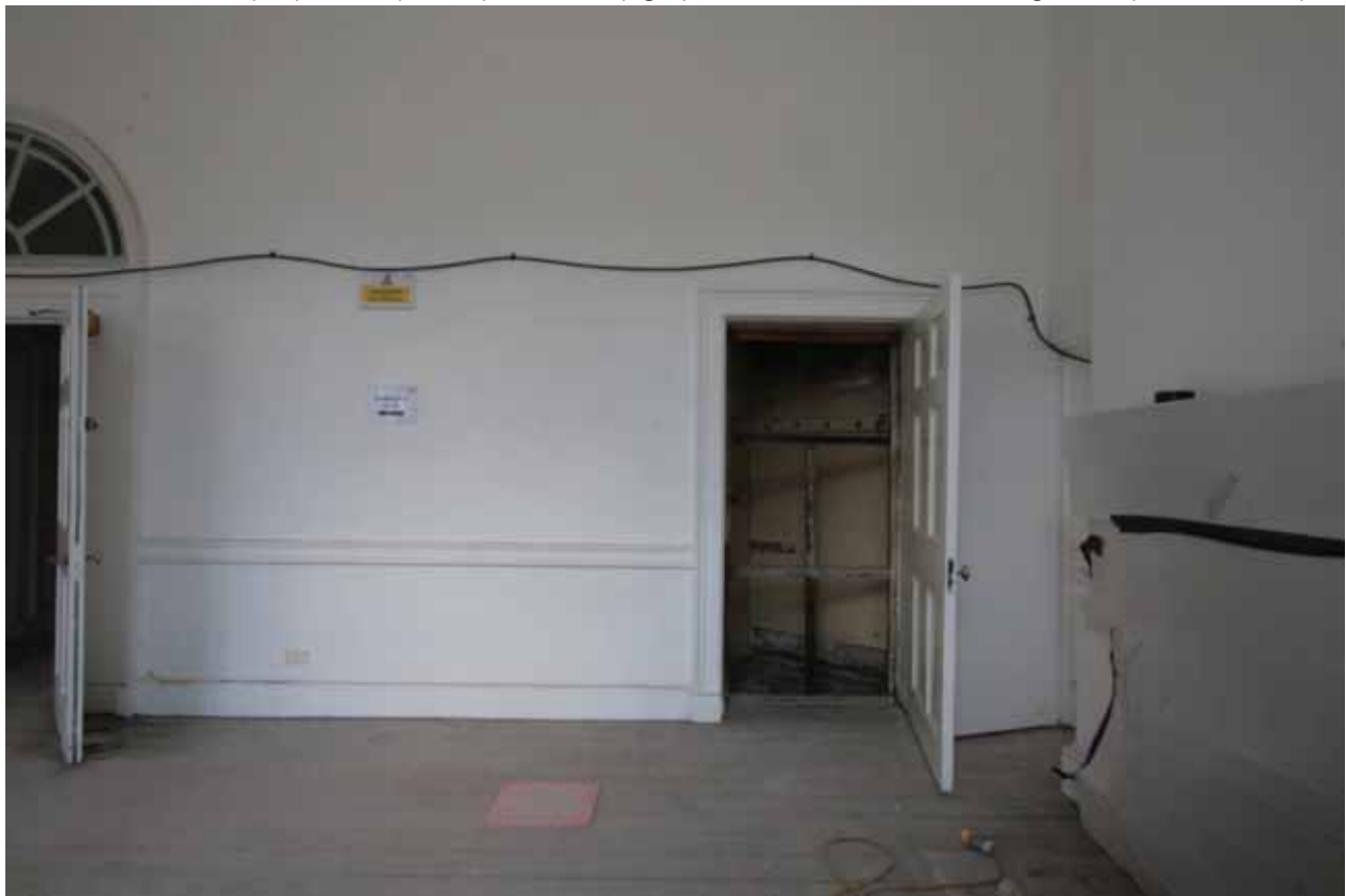
Plate 355: East (left and centre) and south (right) walls in Room G03, looking east (EAF10 275)
