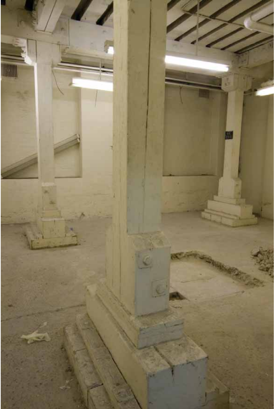
Plate 31: Second World War timber shoring in Rooms B47A, looking north-west (EAF10 D100 029)
