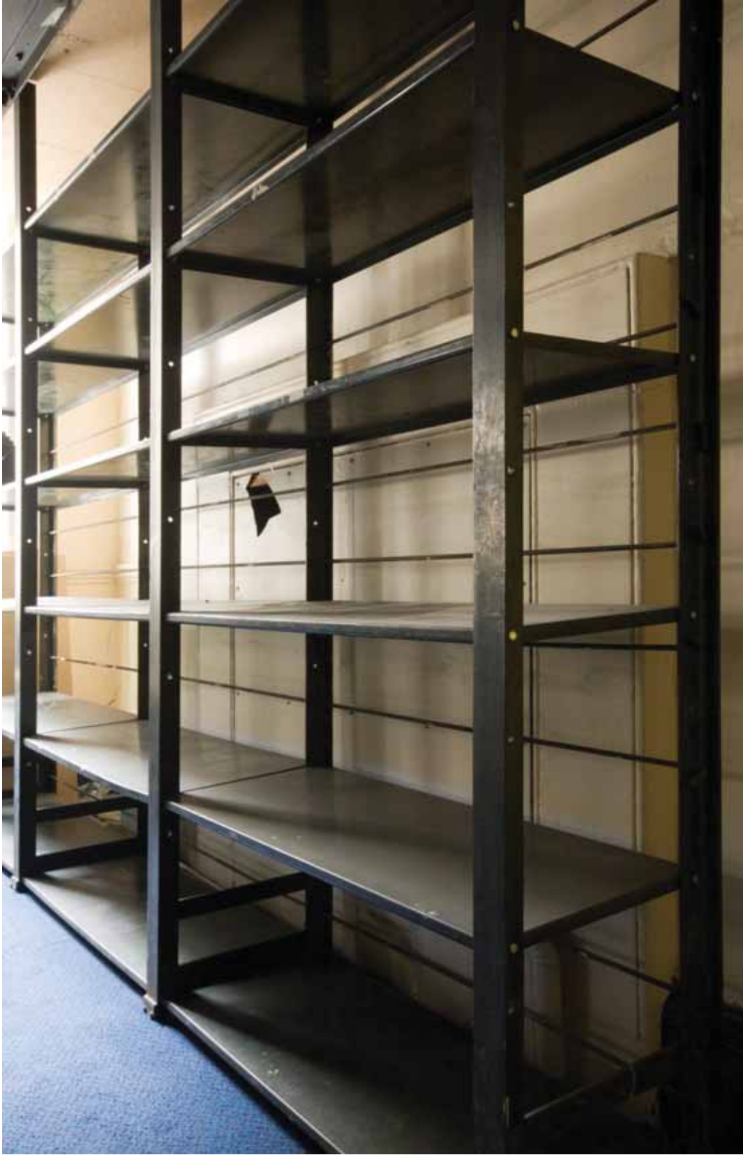
Plate 312: Shelving in front of the south wall in Room M28, looking south-east (EAF10 LG100 0994)
