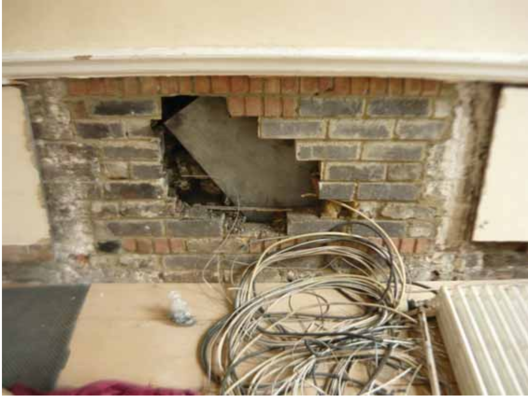
Plate 516: Blocked fireplace in the north wall of Room F64, looking north (EAF10 BHD2 (46))
