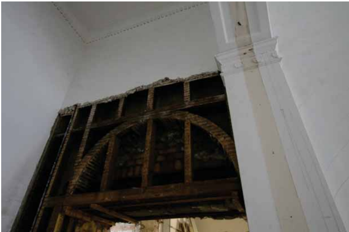
Plate 403b: Area of removed lath and plaster above doorway at the west end of the north wall in Room G38, looking north-west (EAF10 A-D101 008)
