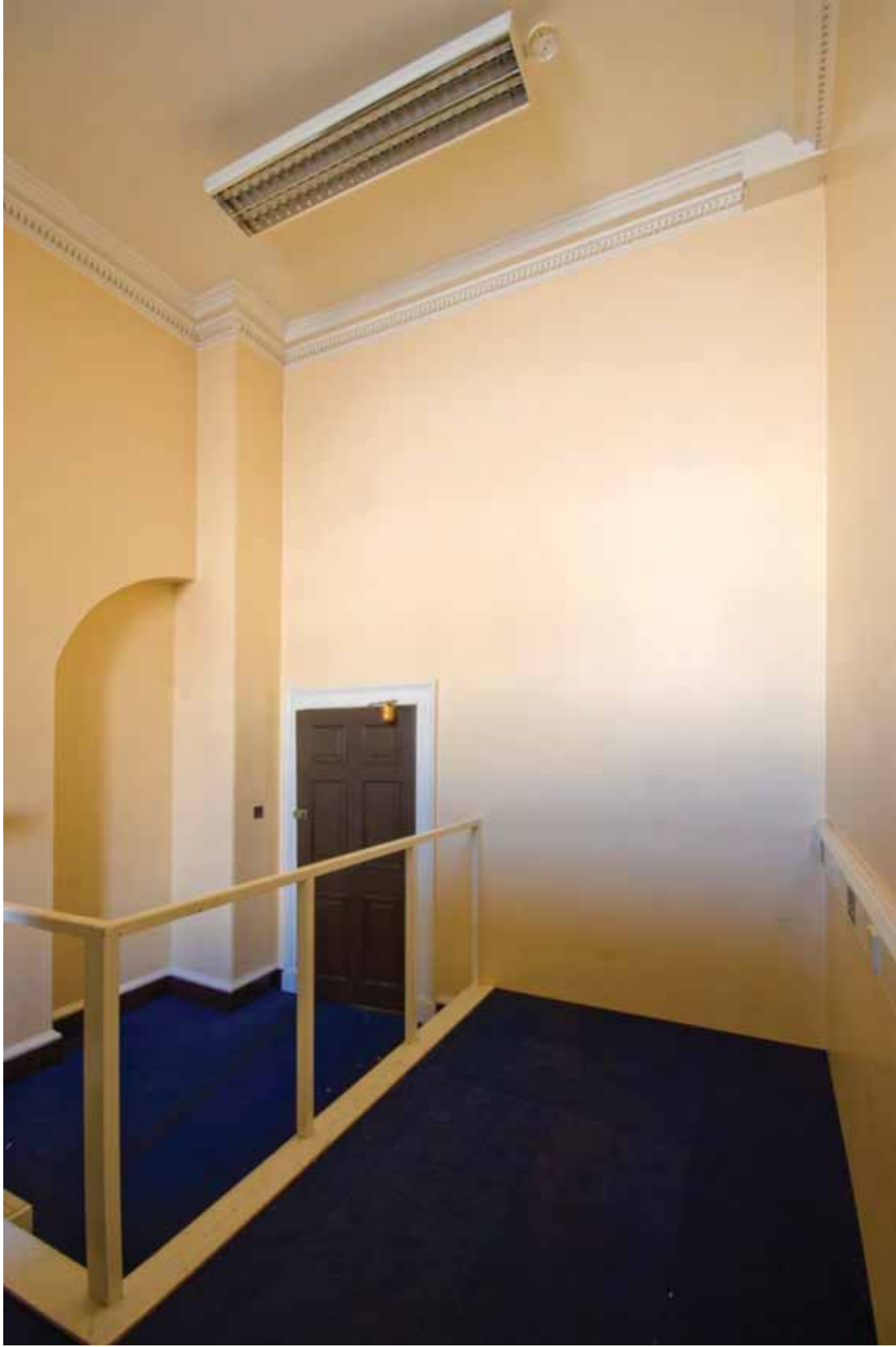
Plate 362: North (left), east (centre) and south (right) walls of Room G04, looking east (EAF10 B100 0907)
