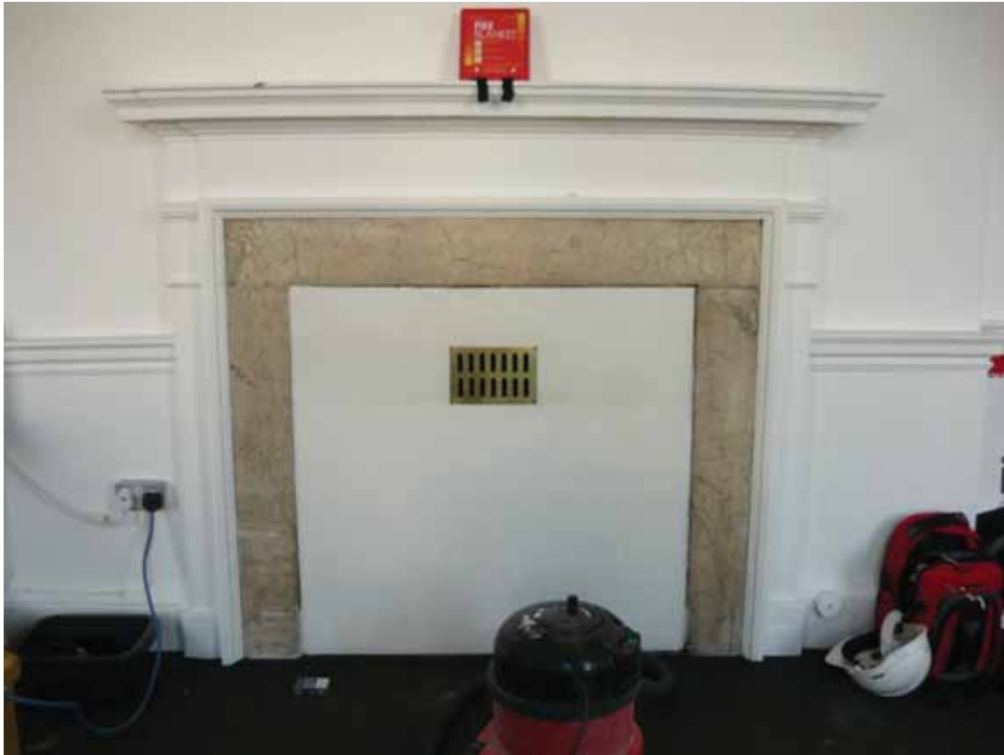
Plate 372: Fireplace in the east wall of Room G09, looking east (EAF10 BHD1 (35))
