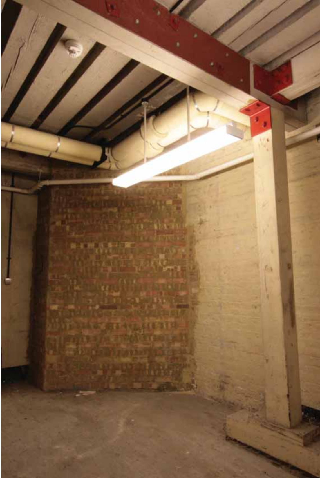
Plate 134: Twentieth century brick partition in the north-west corner of Room B51, looking north-west (EAF10 D100 010)
