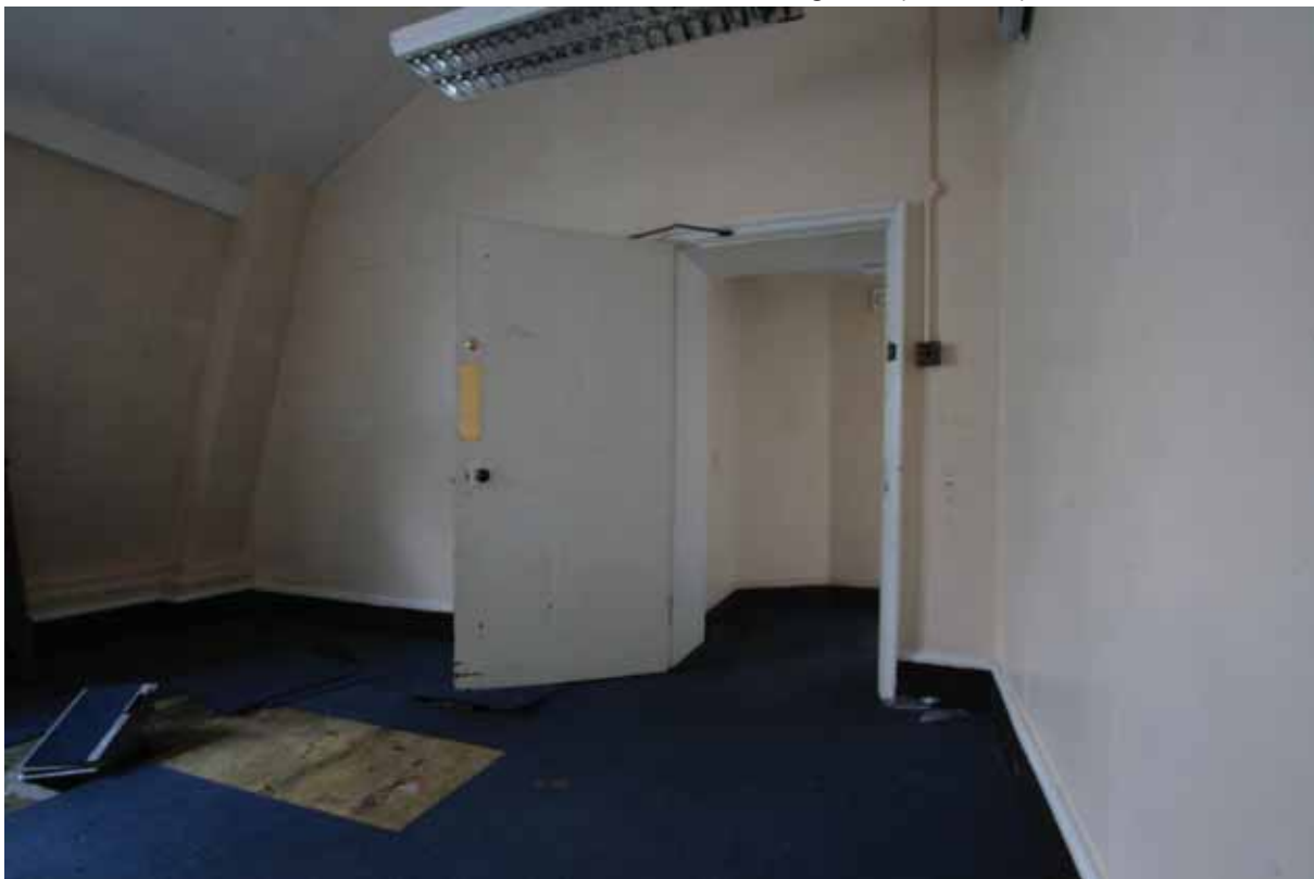
Plate 702: North (left), east (centre) and south (right) walls in Room T14, looking east (EAF10 5a)
