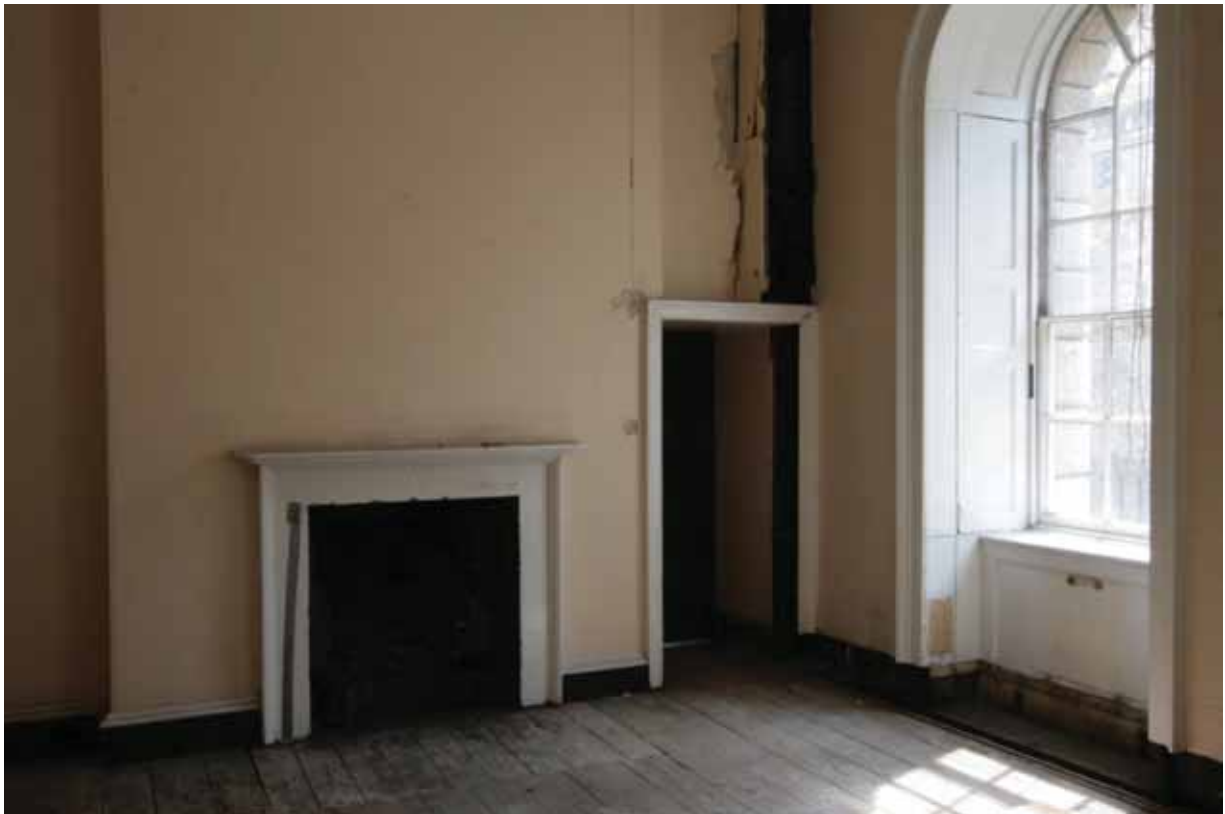
Plate 178: South (left) and west (right) walls of Room M09, looking south-west (EAF10 306)
