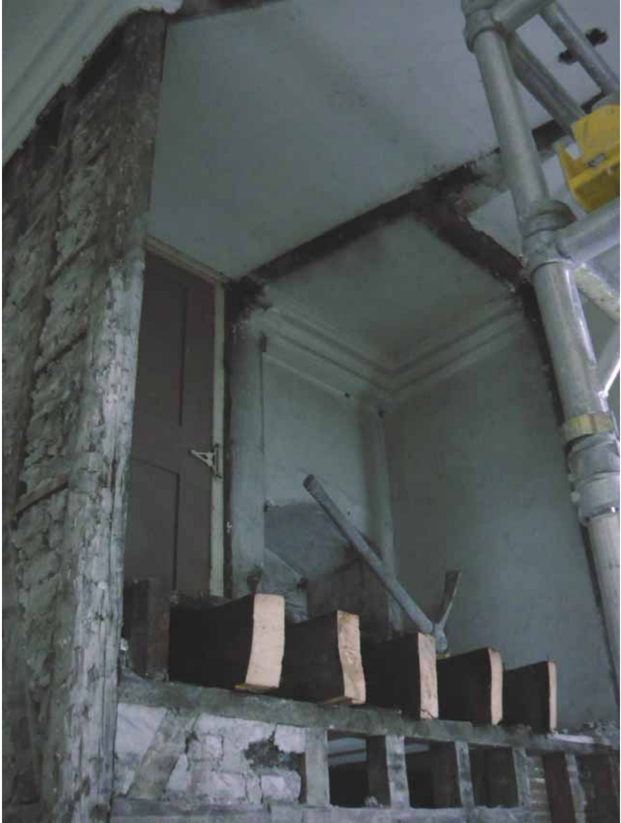
Plate 216: Upper part of the east (left) and north (centre and right) wall of rectangular (in plan) construction in south-west corner of Room M18, looking south-west (EAF10 BHD6 (27))
