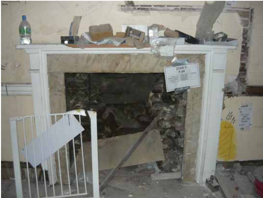
Plate 538: Fireplace (type 11) in the north wall of Room F24, looking north (EAF10 BHD12 (13))
