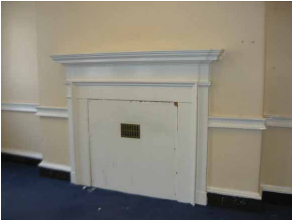
Plate 543a: Fireplace (type 6) in the south wall of Room F26, looking south-east (EAF10 BHD1 (76))
