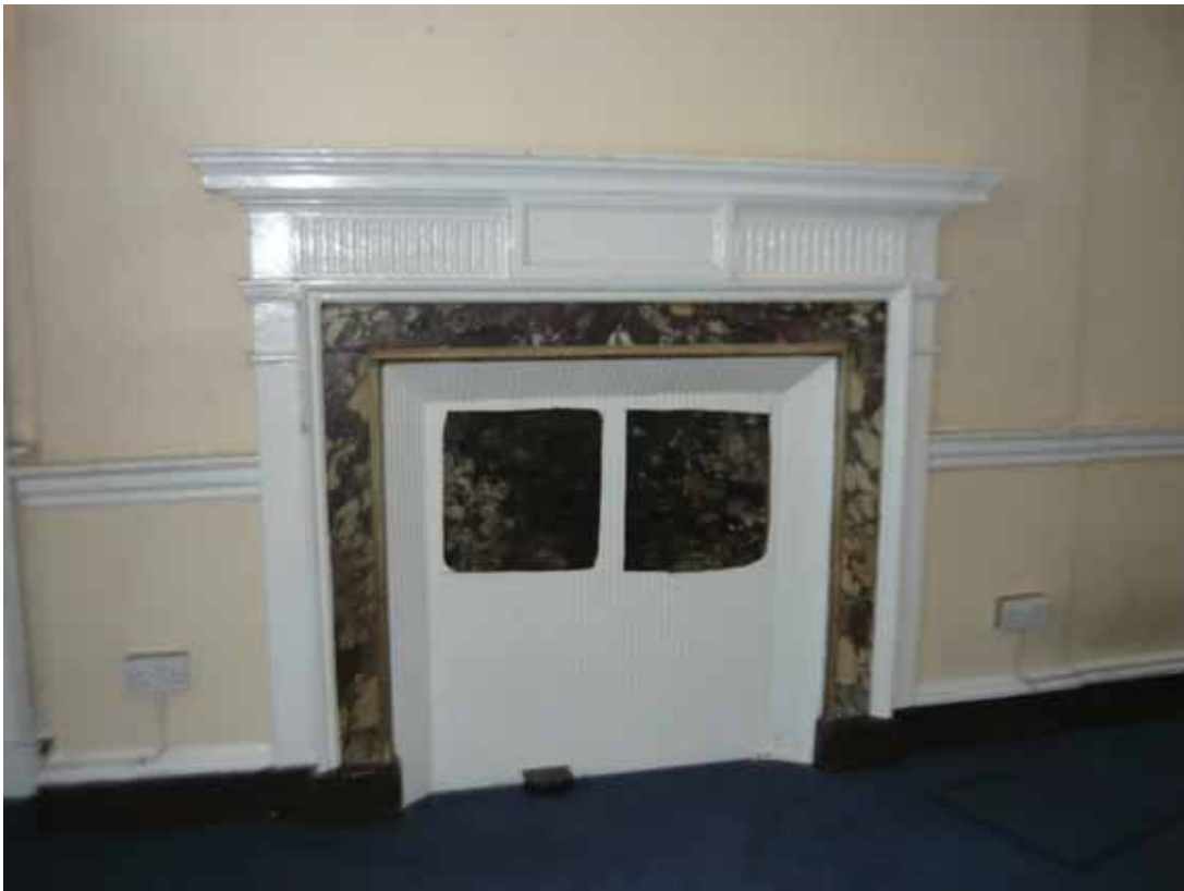
Plate 526: Fireplace (type 7) in the south wall of Room F16, looking south (EAF10 A100 020)
