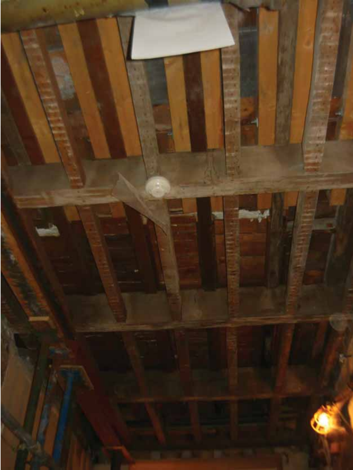
Plate 24b: Primary and secondary floor joists visible following the removal of the lath and plaster ceiling in Corridor next to Rooms B45 and B46, looking west (EAF10 BHD5 (198))
