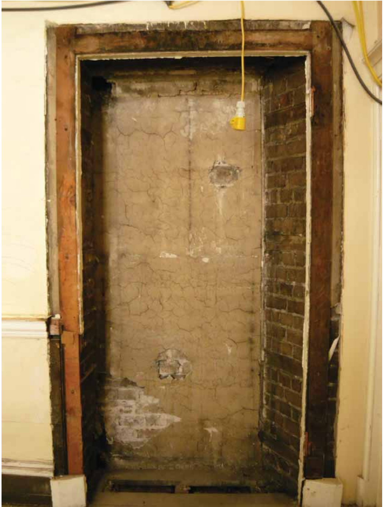
Plate 473: Cupboard at the south end of the east wall in Room F03, looking east (EAF10 BHD8 (23))
