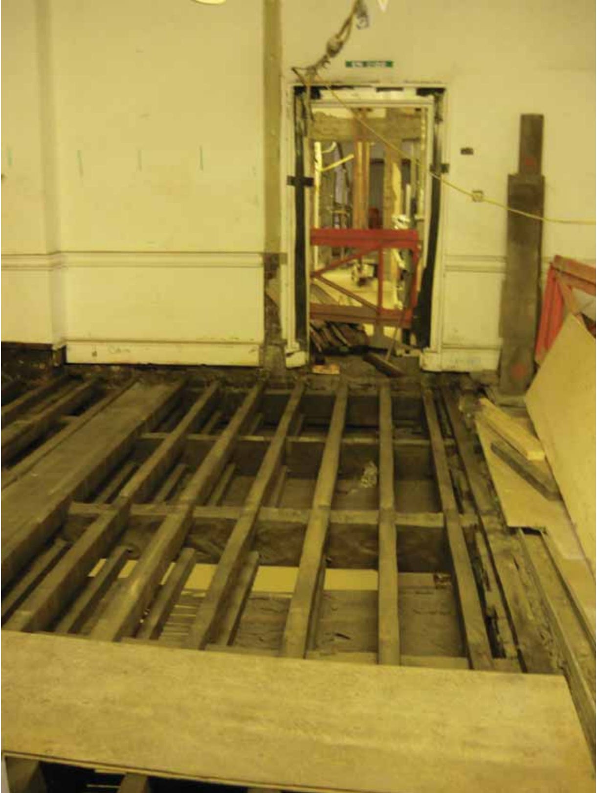
Plate 391b: South wall of Room G16 (left of partition scar) and Corridor 07G (right of partition scar) looking south (EAF10 BHD8 (120))
