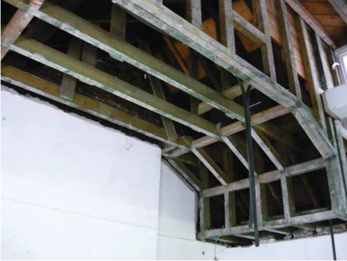
Plate 740: Roof structure above the west wall of Room T118, looking south-west (EAF10 BHD10 (32))
