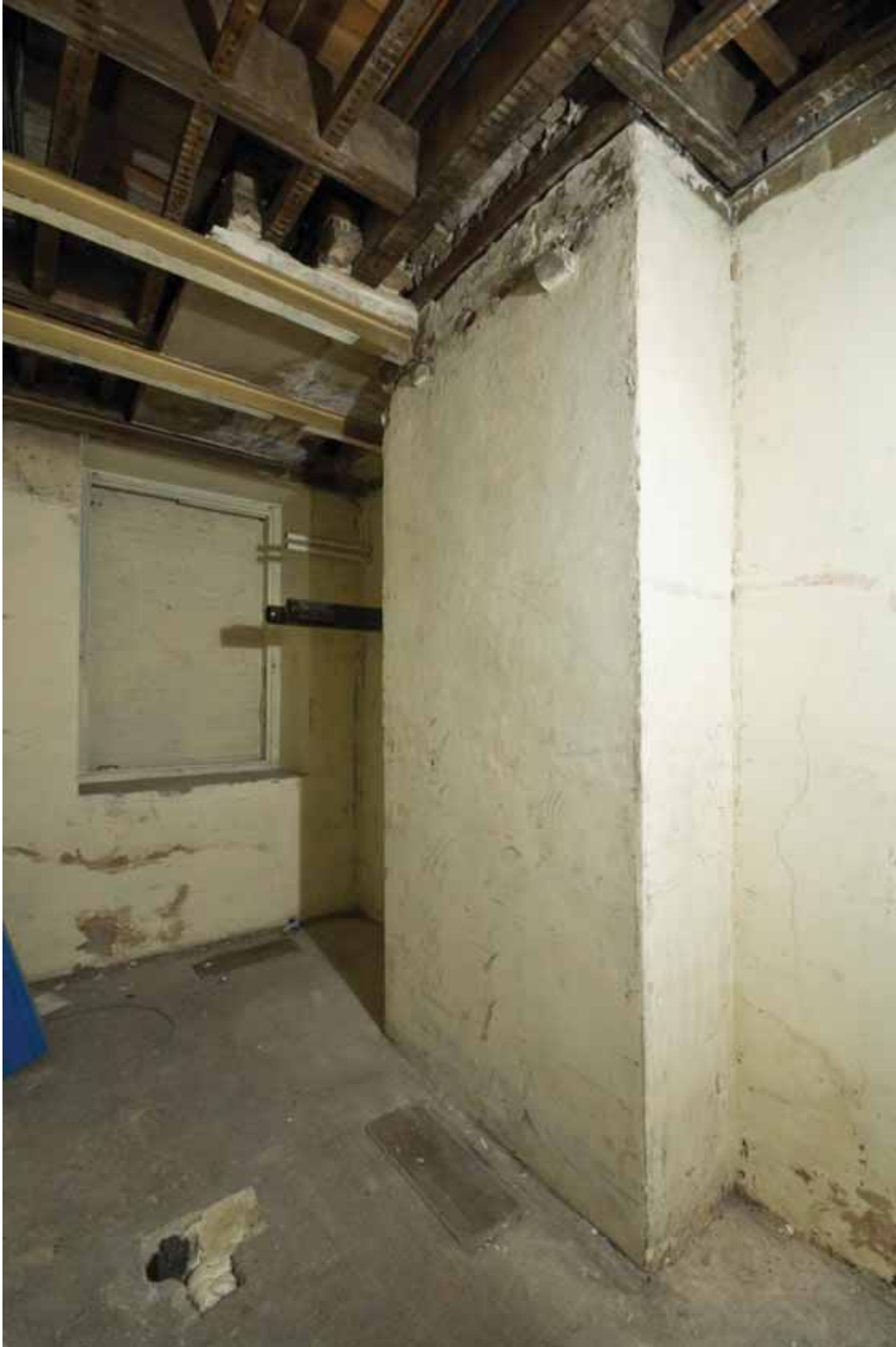
Plate 162: East (left) and south (right) walls of Room B55, looking south-east (DSC_1514 _sitecode EAF10_© PCA Ltd 2010 _1)
