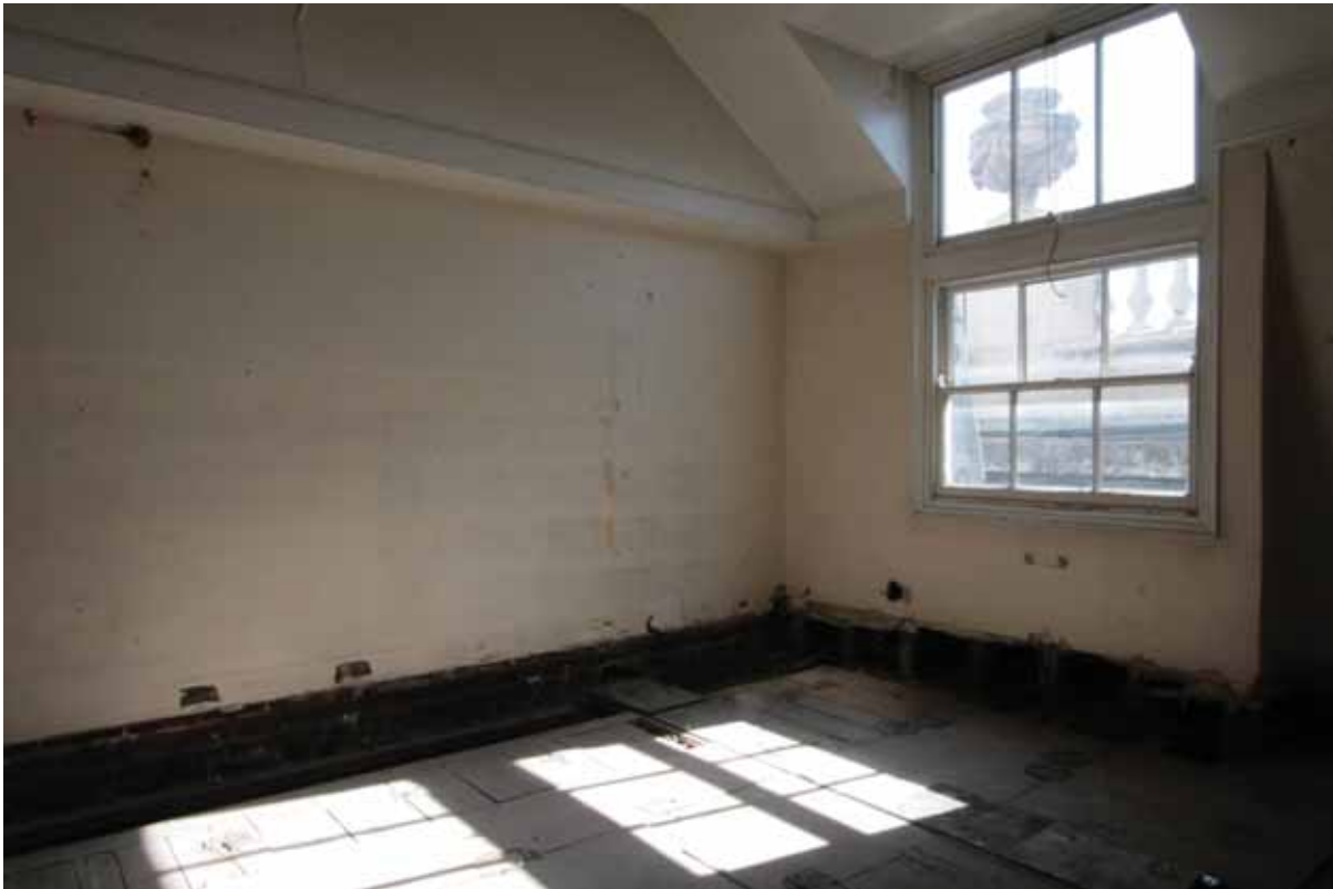
Plate 682: South (left) and west (right) walls of Room T05, looking south-west (EAF10 210)
