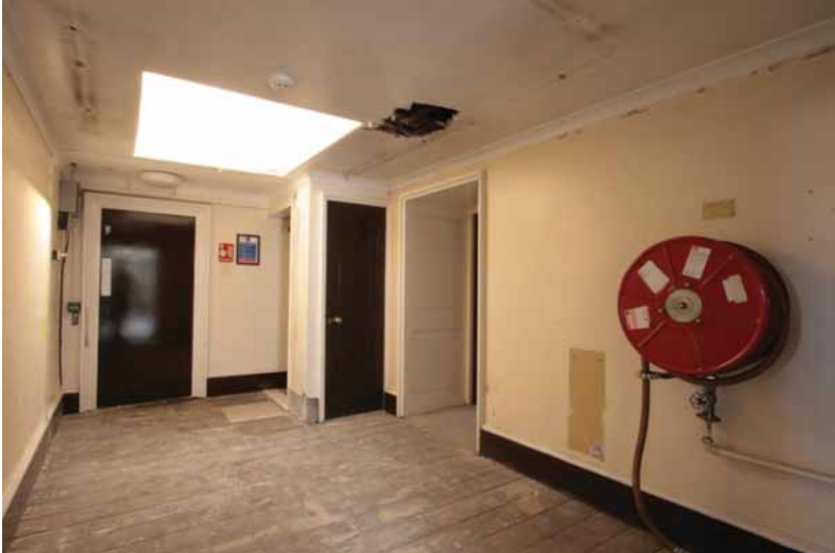
Plate 725: East partition (left), south (left and centre), south partition (centre and right) and north (right) walls in Corridor 10T, looking north-west (EAF10 207)
