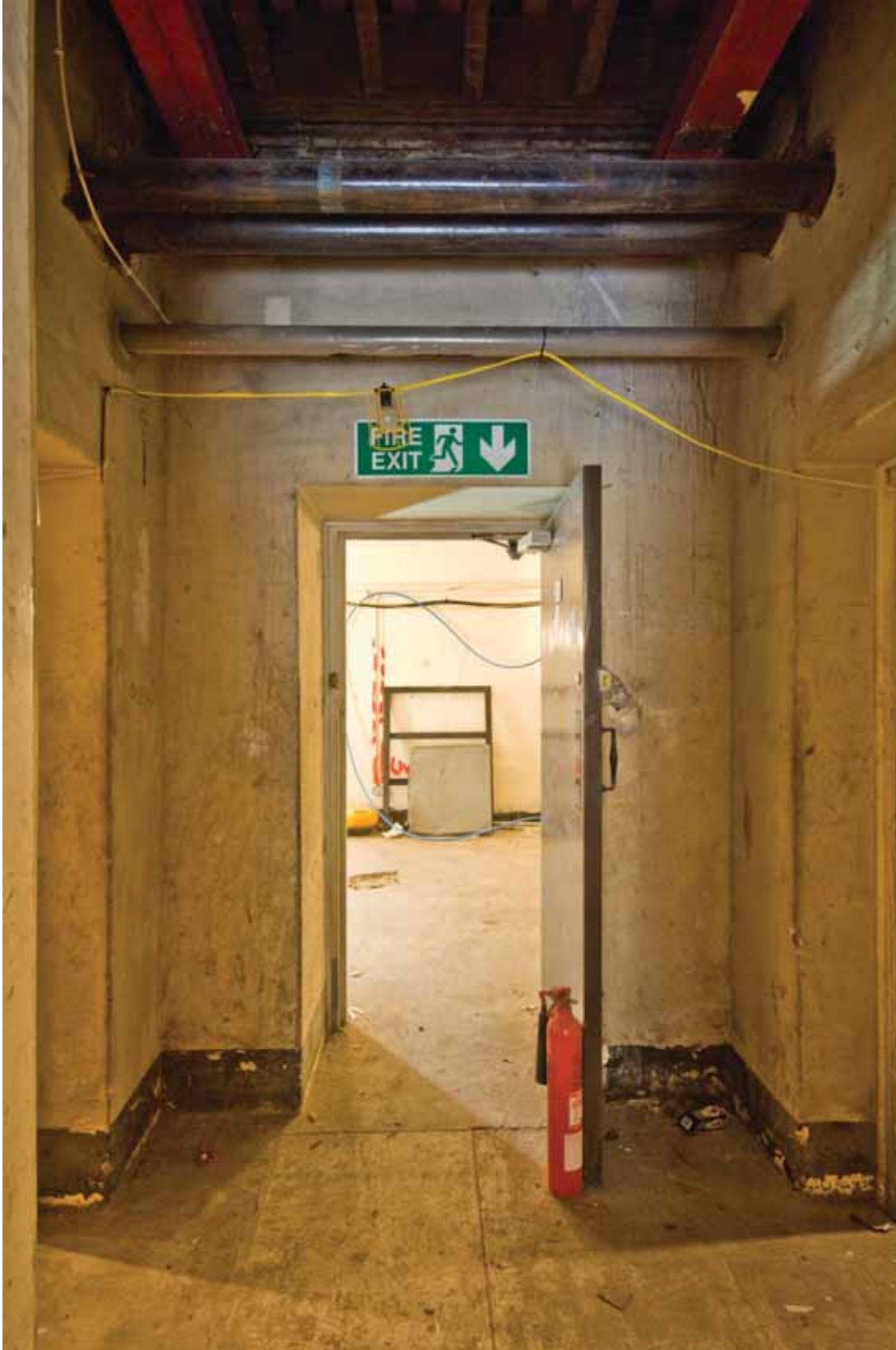
Plate 168: Doorway in the wall of Room B54C, looking west (DSC_1503 _sitecode EAF10_© PCA Ltd 2010 _2)
