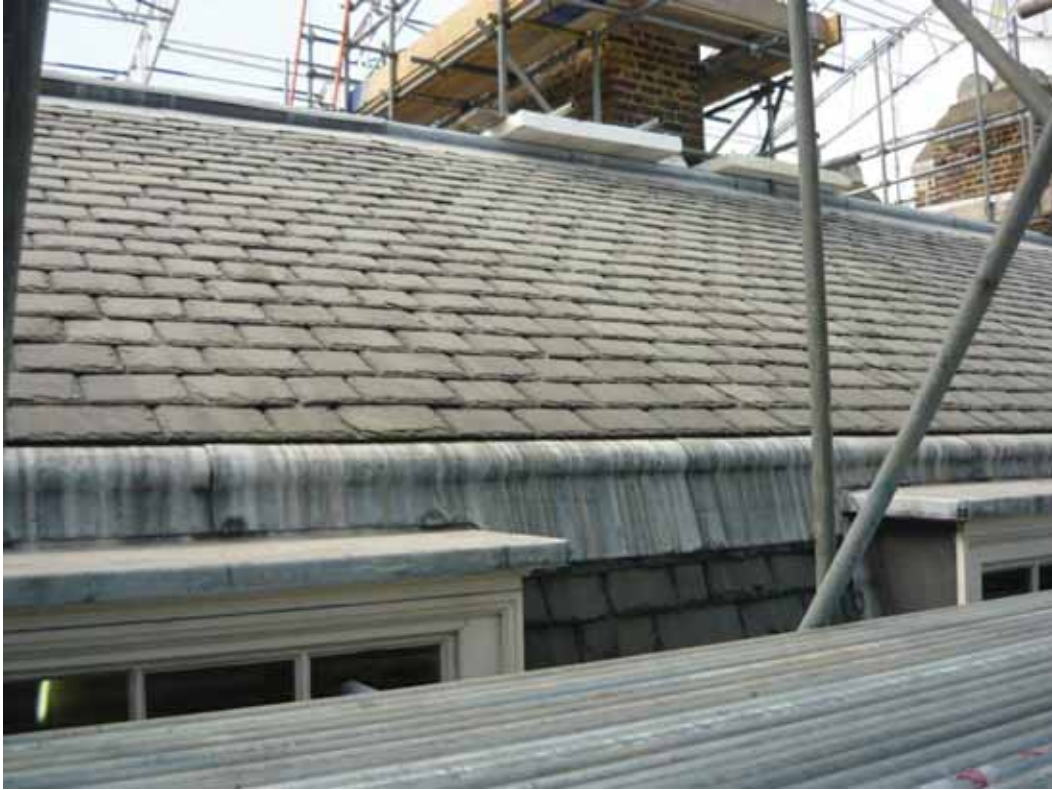
Plate 806: Tops of Room T24's sash windows in the east wall of the East Wing at third floor level, looking north-west (EAF10 BHD9 (9))
