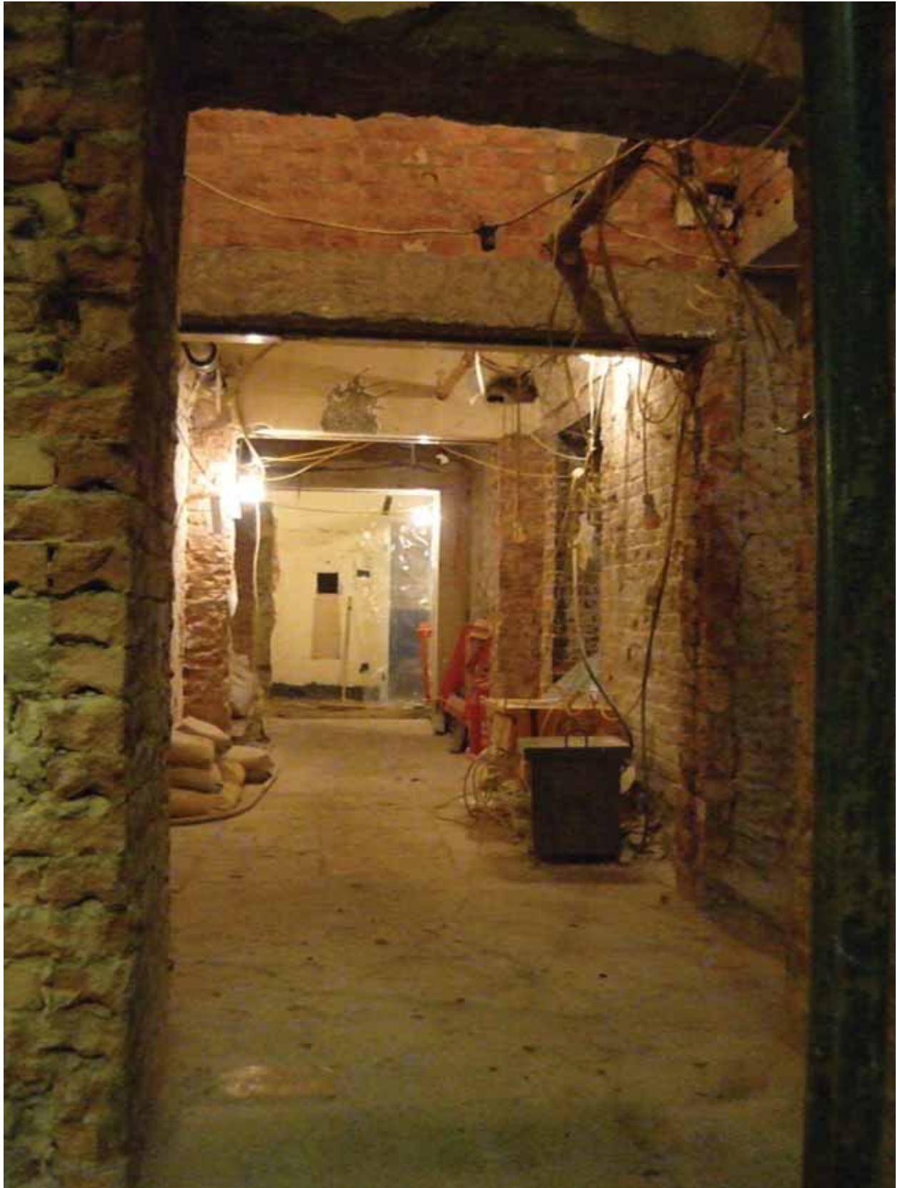
Plate 80: View south from Stairs 01 to Corridors 1A, 1B, 1C and 1D (EAF10 BDH6(57))
