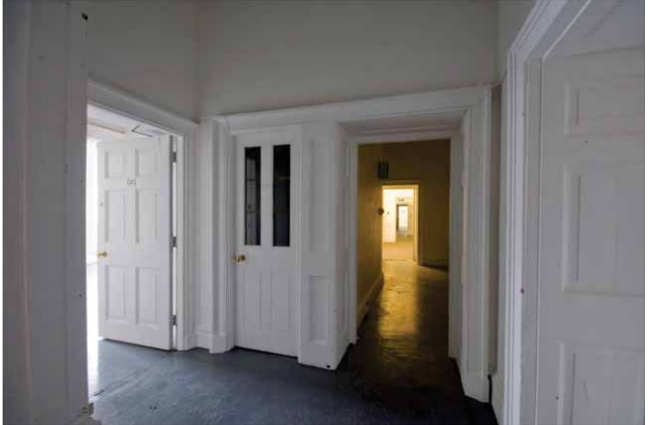
Plate 397: West (left) and north (centre) walls of Cupboard 02G, looking north-west (DSC_0824 sitecode EAF10 © PCA Ltd 2010)
