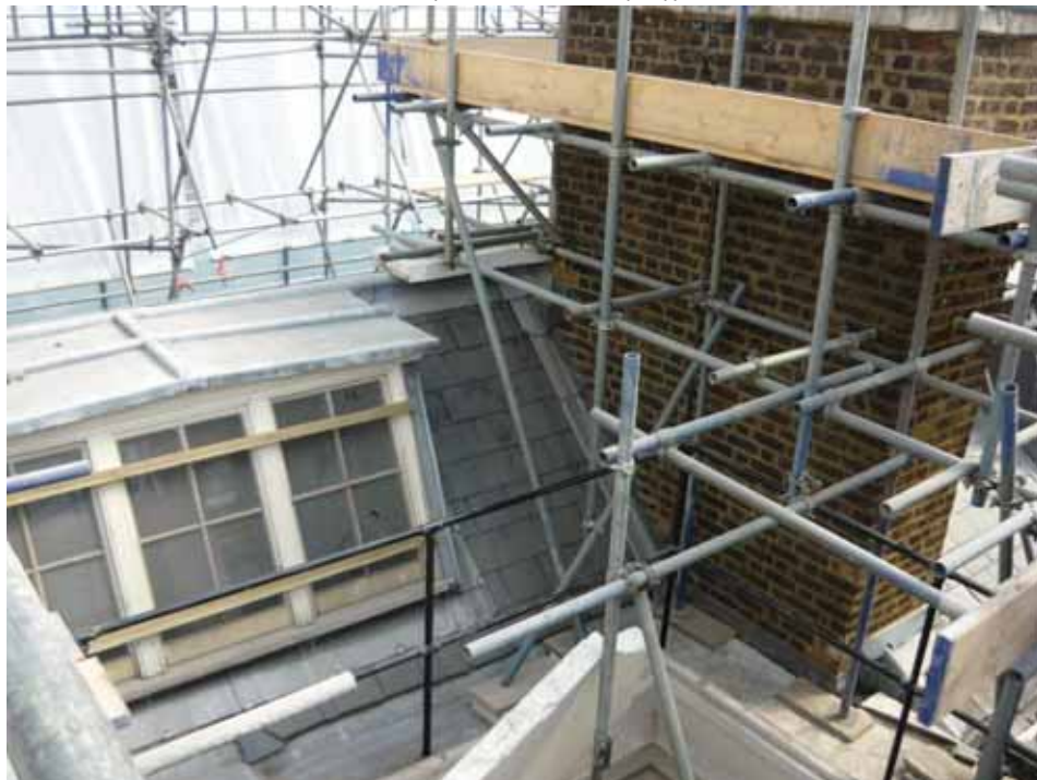
Plate 804: Dormer window over Room T25 and chimney stack between Rooms T24 and T25, looking south-east (EAF10 BHD9 (5))
