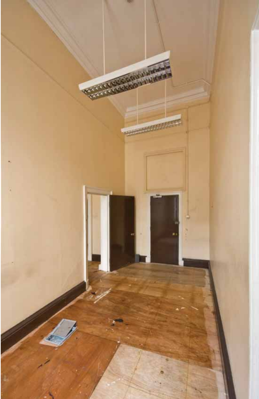
Plate 299: South (left), east (centre) and north (right) walls in Room M26, looking west (EAF10 LG100 1008)
