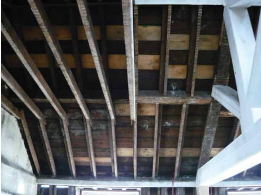
Plate 747: North end of the east side of the roof above Room T15, looking east (EAF10 BHD10 (29))
