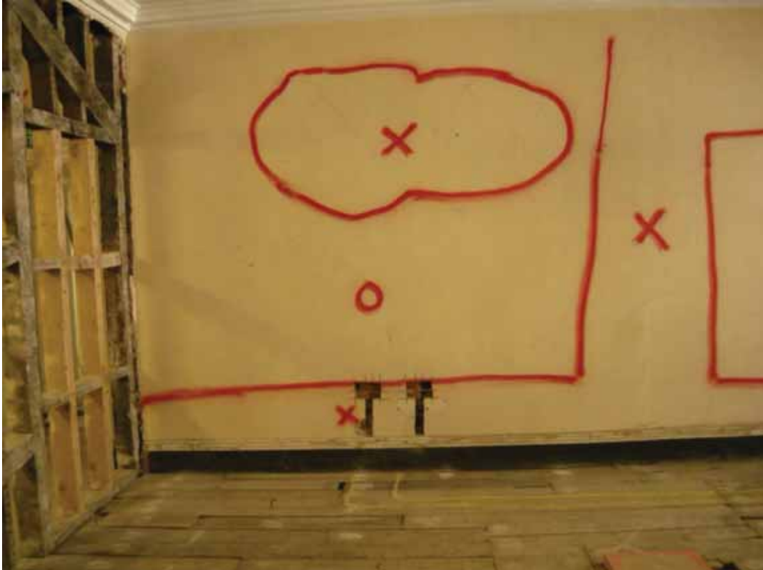
Plate 622: West partition (left) and north (right) walls in Room S16, looking north (EAF10 BHD8 (39))
