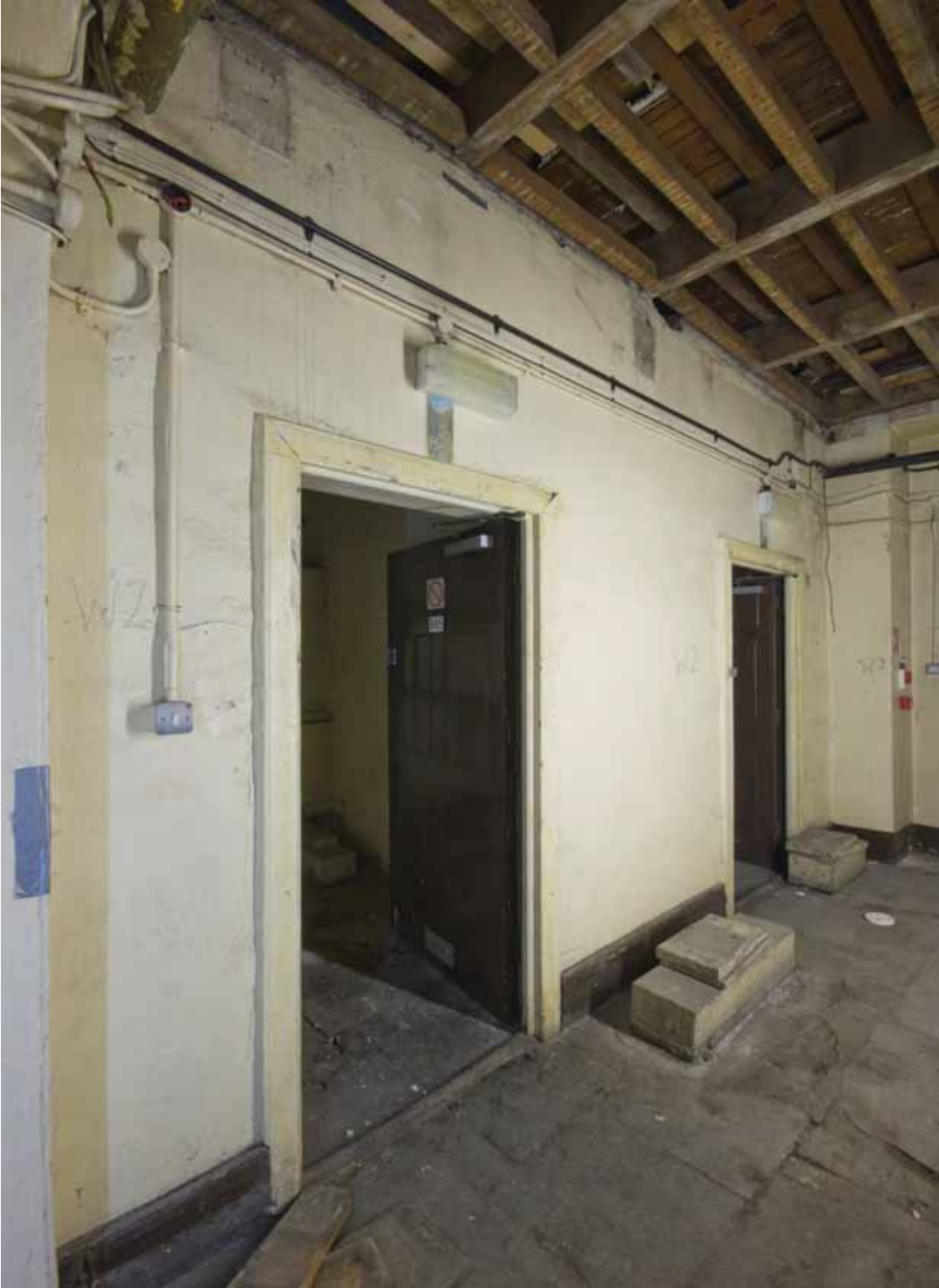
Plate 17: Doorways into Rooms B45 (left) and B46 (right) from Corridor, looking south-west (DSC_1369 _sitecode EAF10_© PCA Ltd 2010)
