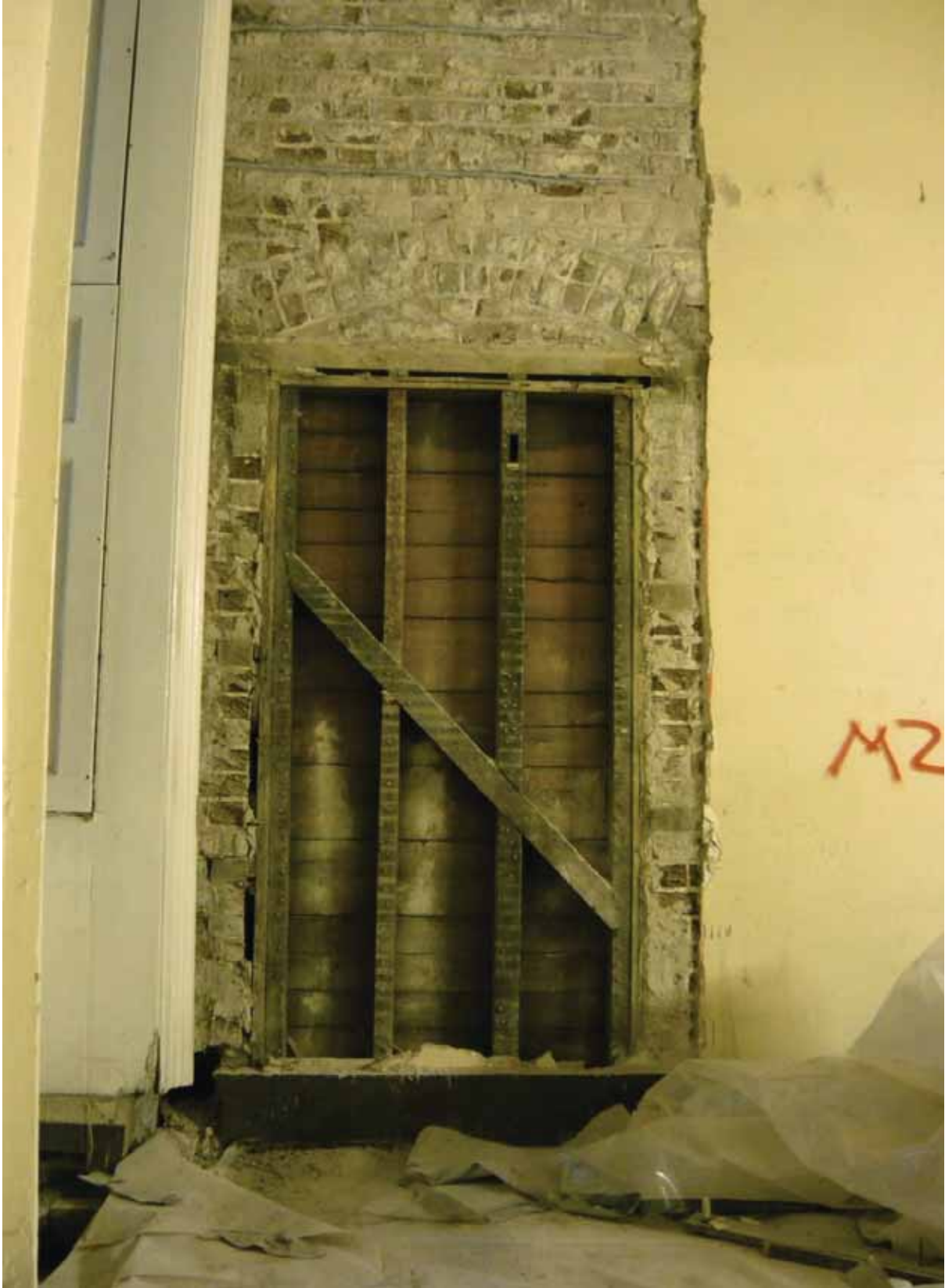
Plate 295: Doorway uncovered at the east end of the south wall in Room M25, looking south (EAF10 BHD6 (82))
