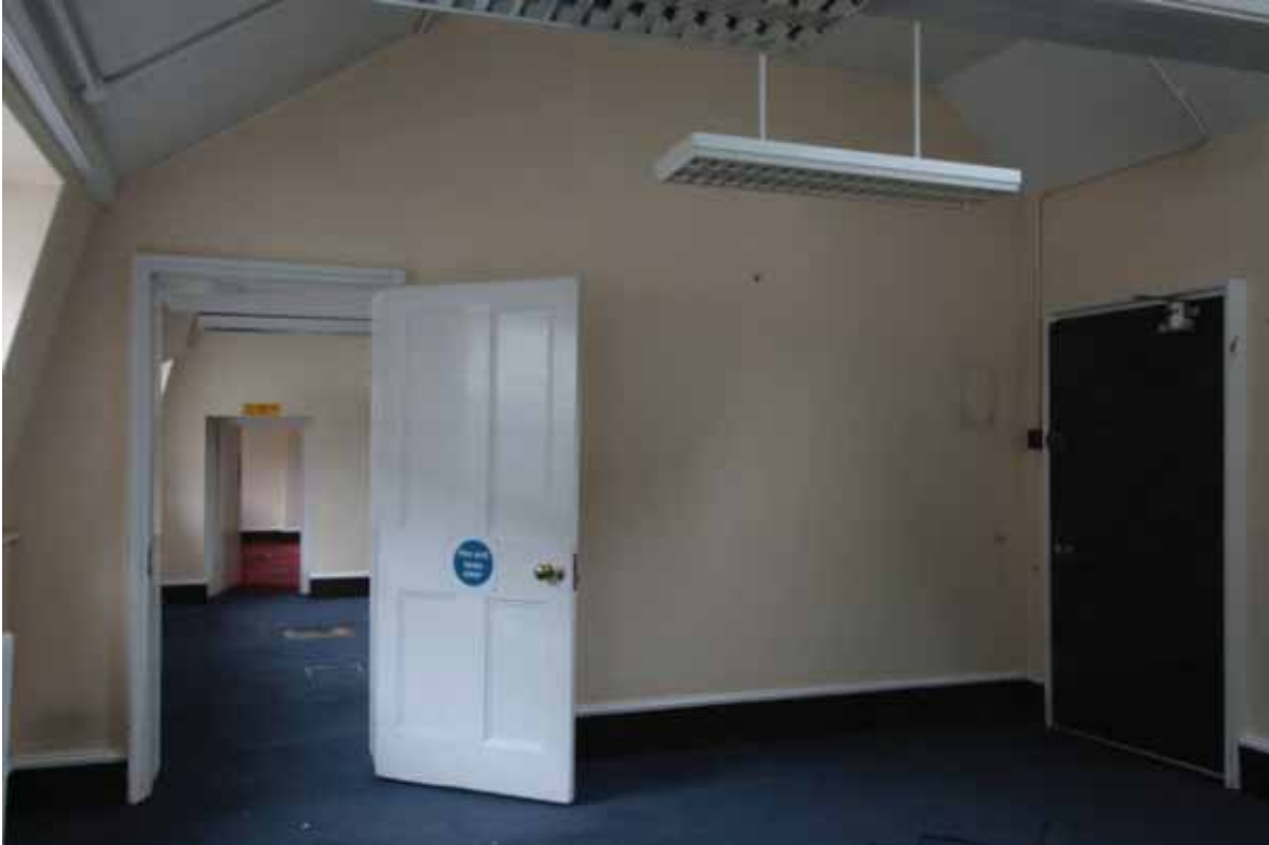
Plate 751: South (left and centre) and west (right) walls in Room T17, looking south (EAF10 45)
