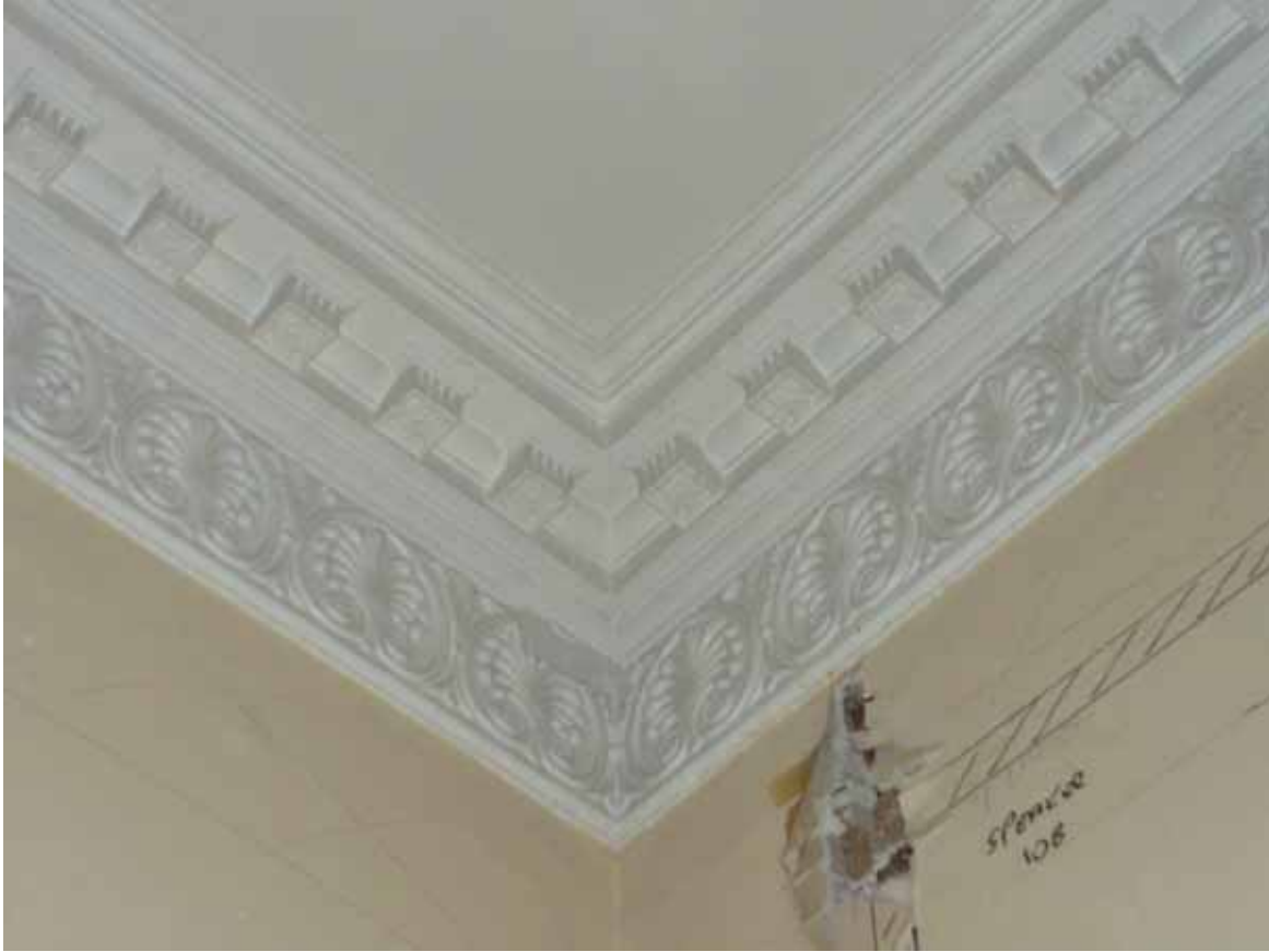
Plate 540: Cornice in the north-west corner of Room F24, looking north-west (EAF10 BHD11 (29))
