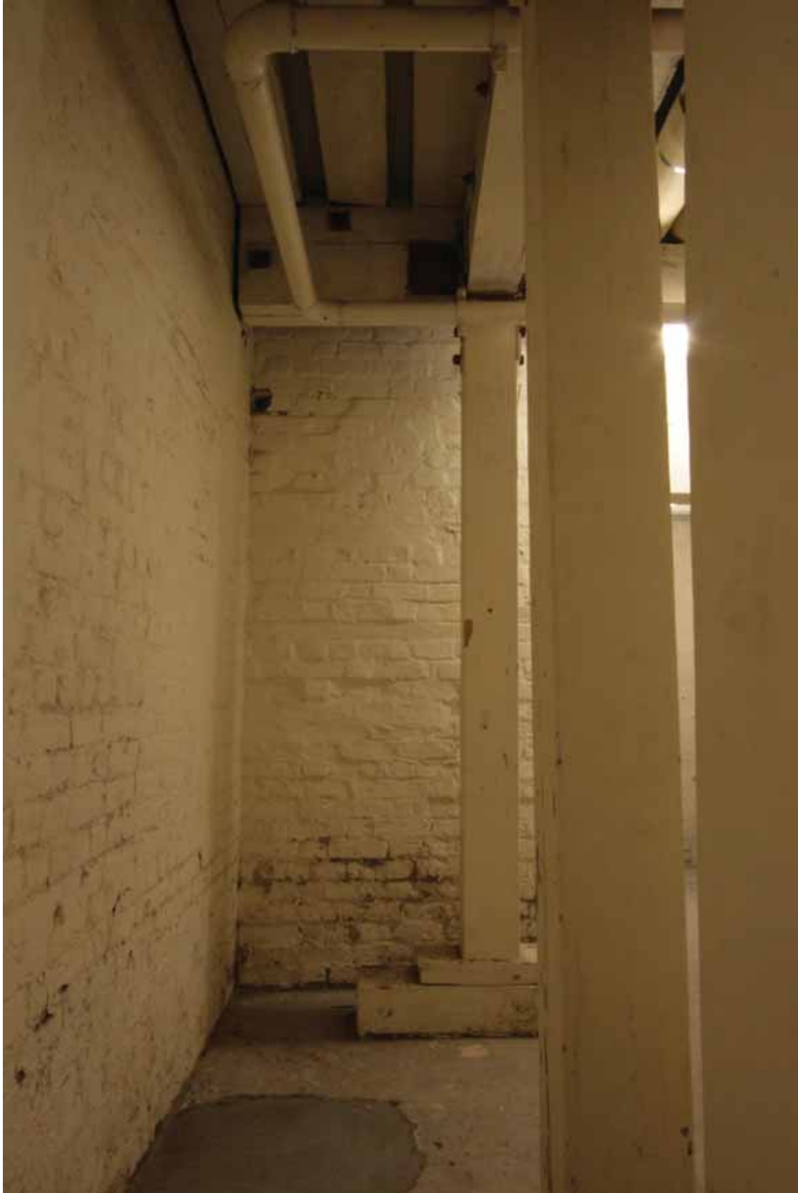
Plate 116: West (left) and north (right) walls of Room B49A, looking north (EAF10 D100 008)
