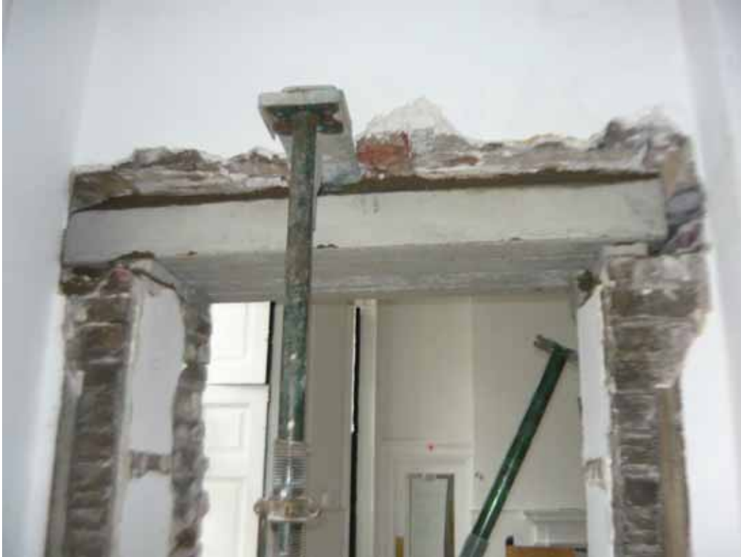
Plate 412: Doorway opened up at the east end of the south wall in Room G16, looking south (EAF10 BHD3 (38))
