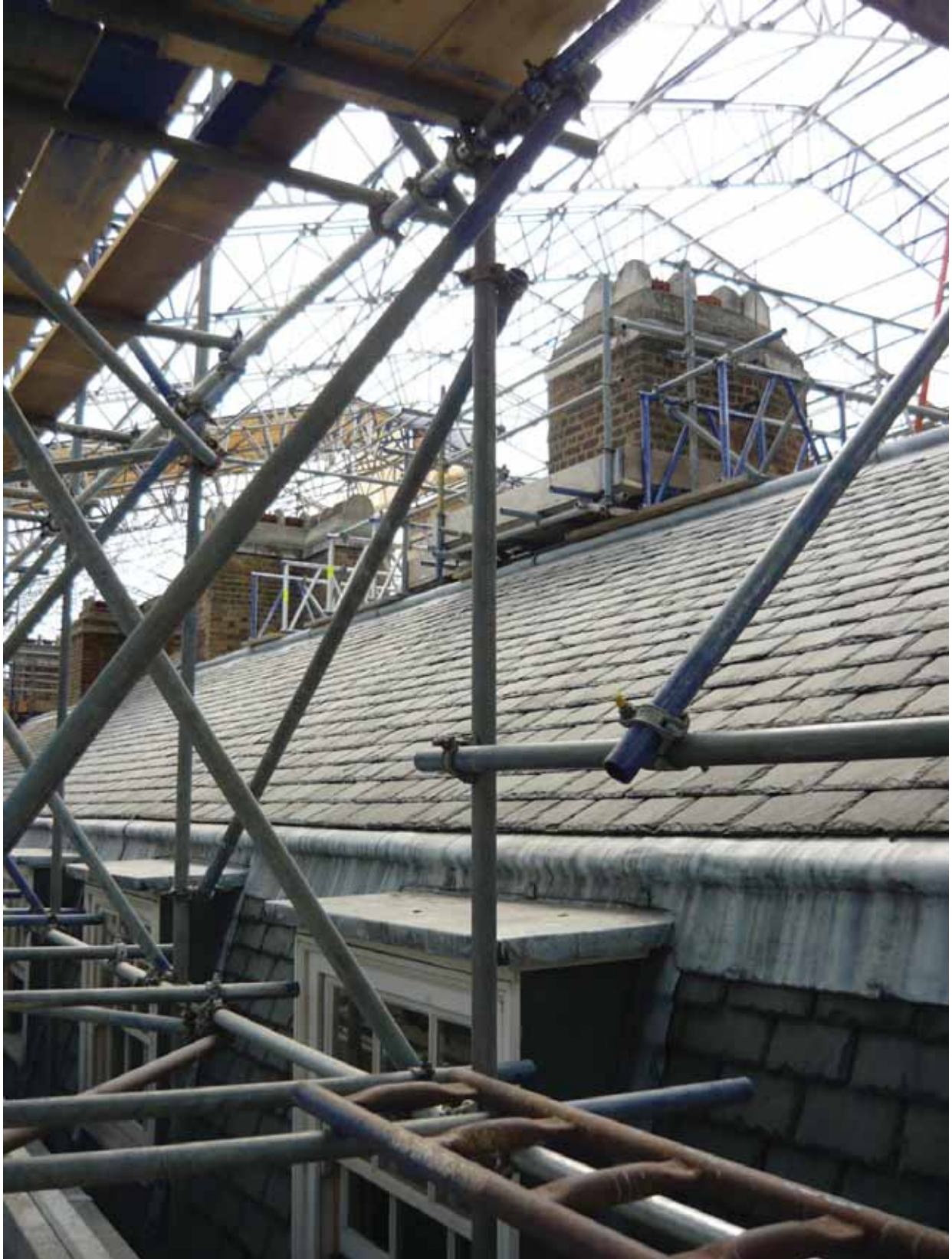
Plate 805: Room T23 sash windows in the east wall of the East Wing at third floor level, looking southwest (EAF10 BHD9 (8))
