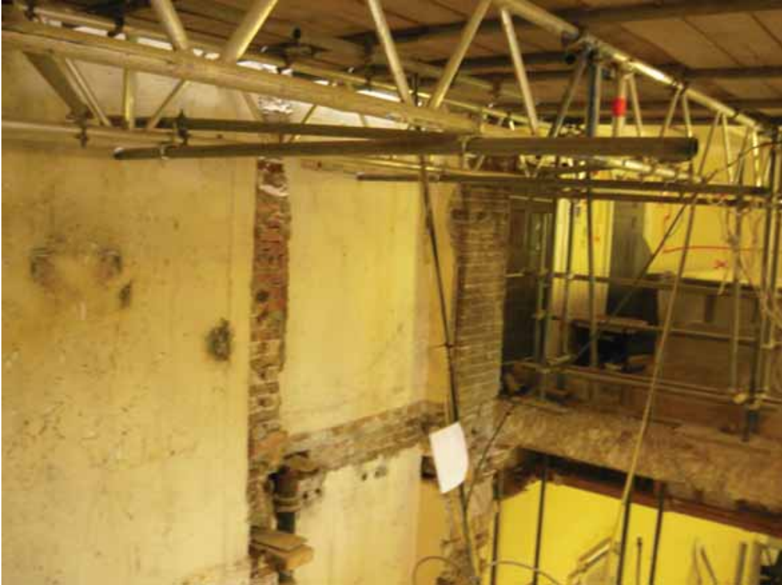
Plate 596: East wall of Lift/Cupboard 01S and Corridor 05S (beyond), looking south-east (EAF10 BHD8 (152))
