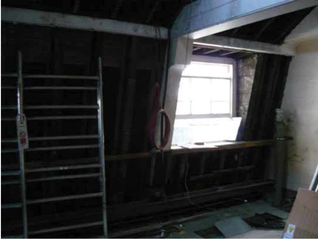
Plate 789: East (left and centre) and south (right) walls in Room T28, looking south-east (EAF10 BHD10 (6))
