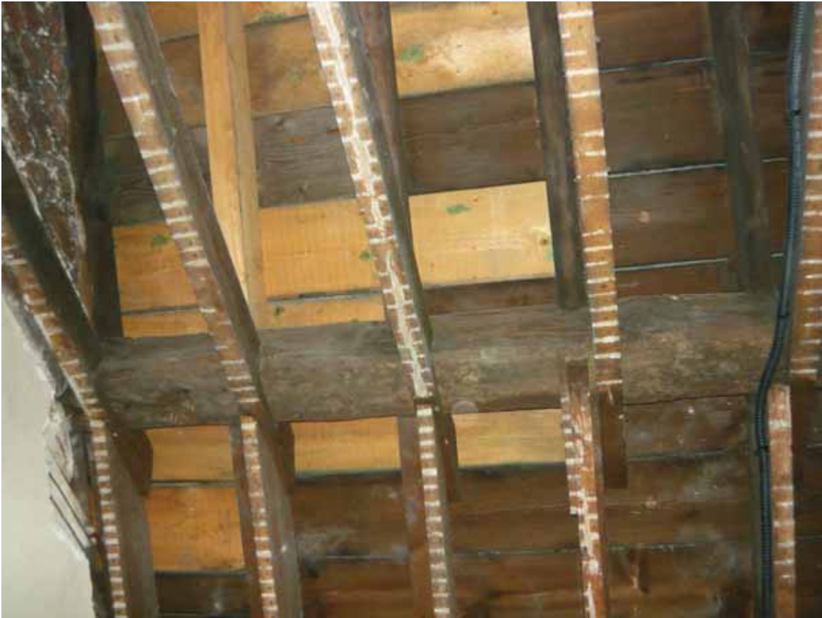
Plate 664: Roof structure at the south end of Room T01, looking west (EAF10 BHD10 (54))
