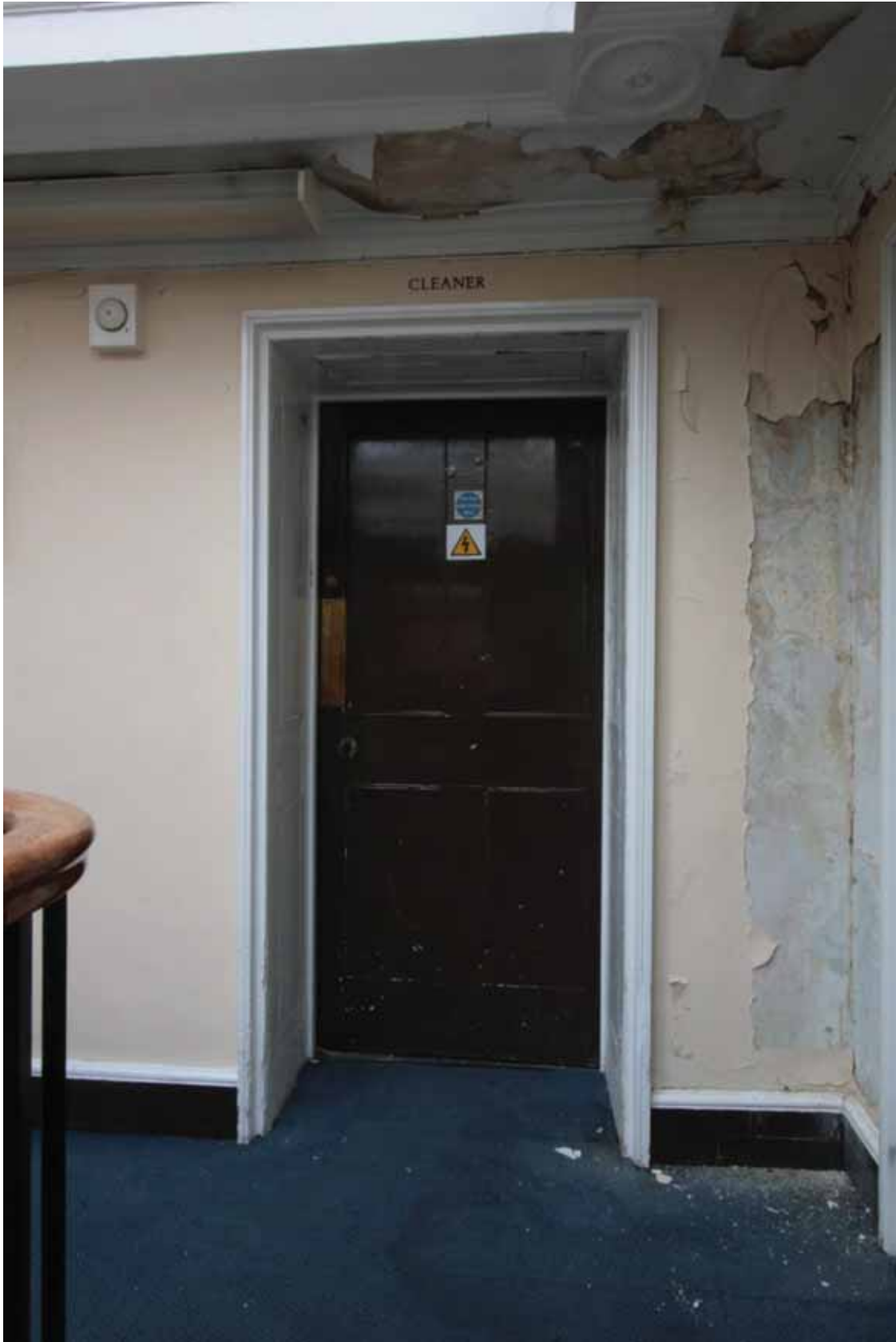
Plate 717: Doorway at the east end of the north wall in Corridor 05T, looking north (EAF10 39)
