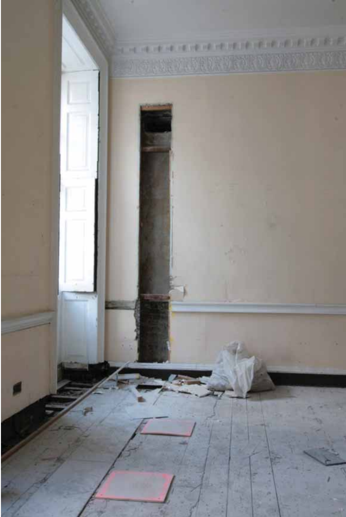
Plate 539: East (left) and south (right) walls in Room F24, looking south (EAF10 261)
