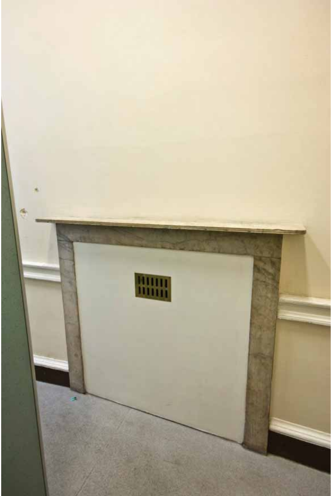
Plate 435: Fireplace (type 15) in the south wall of Room G23, looking south-east (EAF10 B100 0913)
