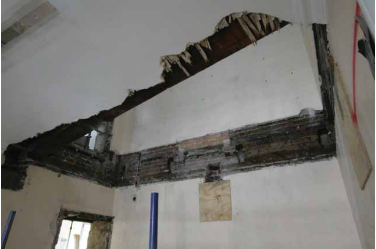
Plate 706: East (left), south (centre) and west (right) walls in Room T14, looking south (EAF10 A100 017)
