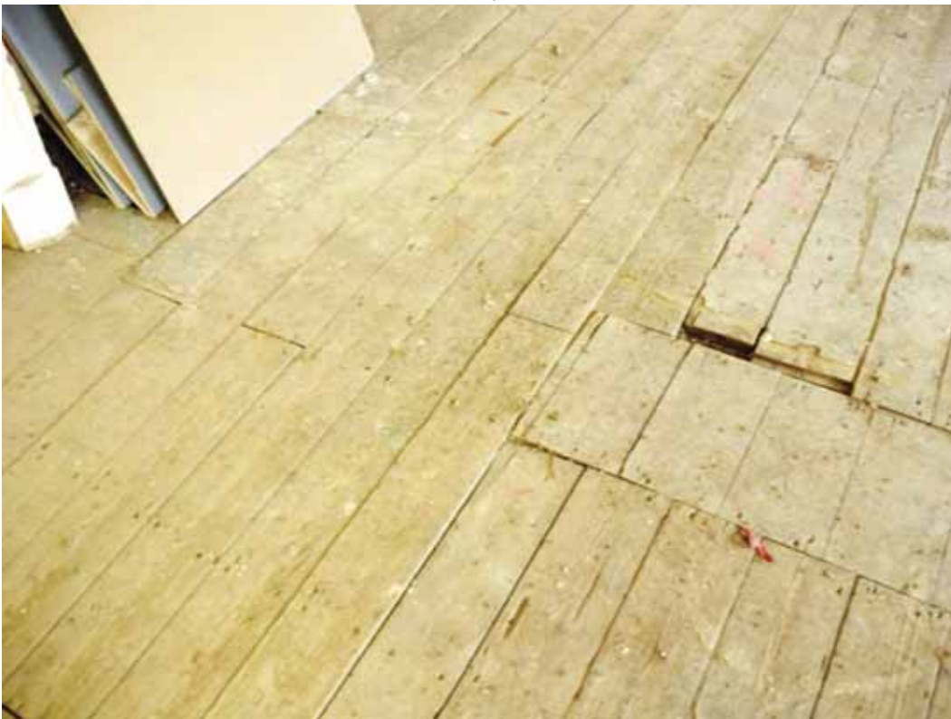
Plate 572: Scar of east-west partition wall in floorboards in Room S08/S09, looking south-east (EAF10 BHD8 (150))
