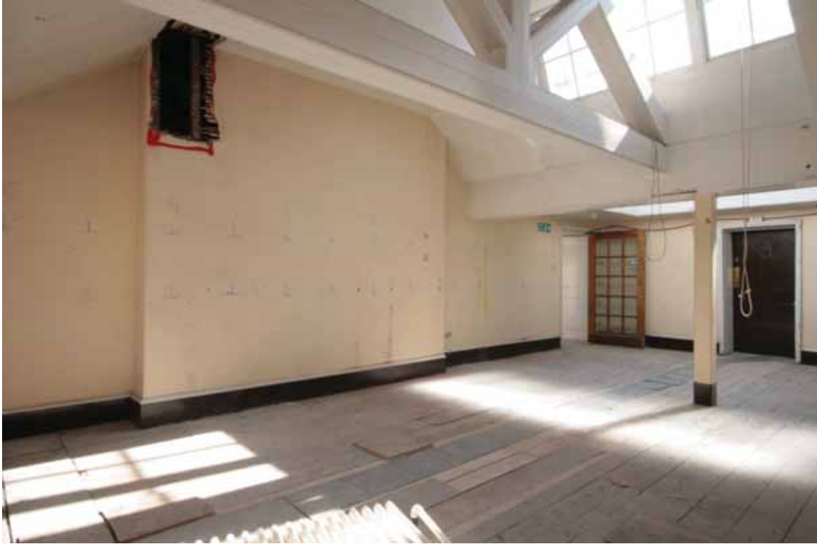
Plate 744: South (left) and west (right) walls in Room T15, looking south-west (EAF10 208)
