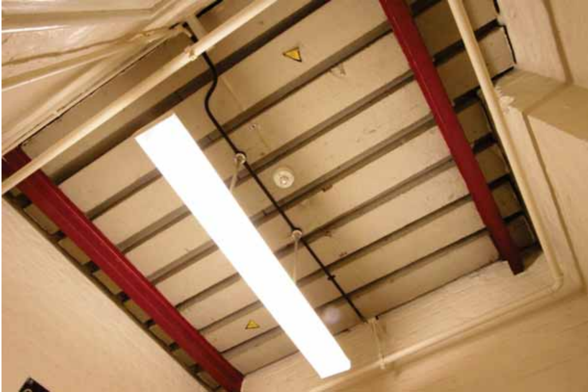
Plate 58: World War 2 rolled steel joists supporting timbers just below the ceiling in Room B48B, looking north (EAF10 D100 039)
