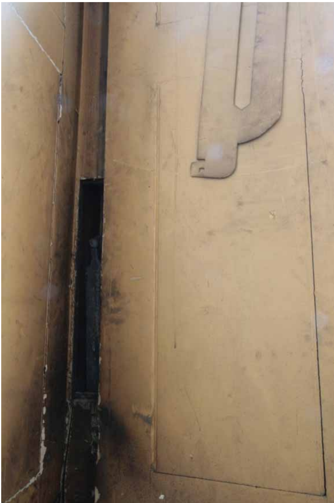
Plate 529: Sash weight for the north window in the east wall of Room F17, looking east (EAF10 258)
