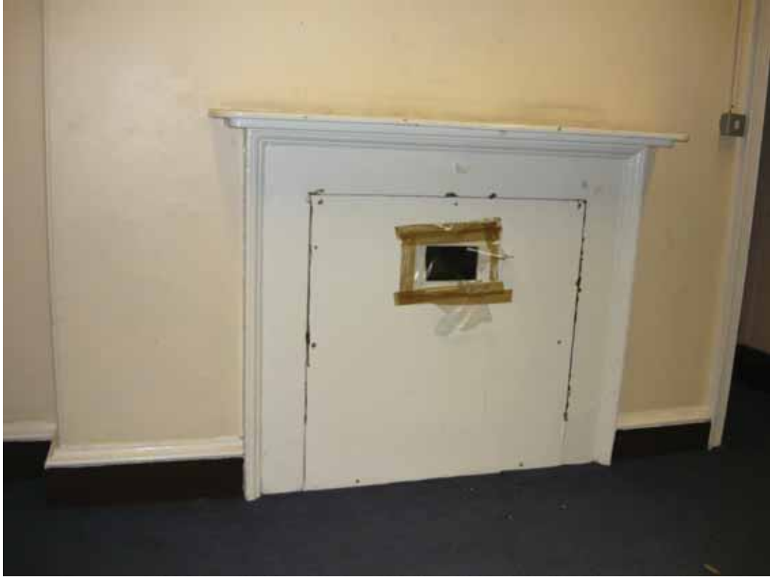
Plate 182: Fireplace in the south wall of Room M09, looking south (EAF10 BHD1 (25))
