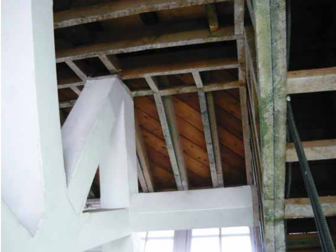
Plate 742: Roof structure above the west wall of Room T118, looking west (EAF10 BHD10 (31))
