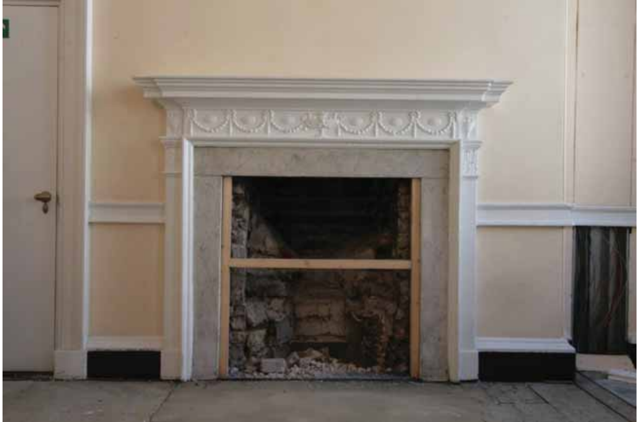
Plate 530: Fireplace (type 9) in the north wall of Room F18, looking north (EAF10 178)
