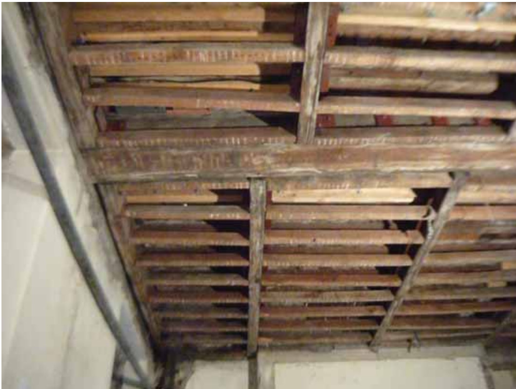
Plate 40: Primary and secondary floor joists visible following the removal of the lath and plaster ceiling in Room B47A, looking north-west (EAF10 BHD5 (87))
