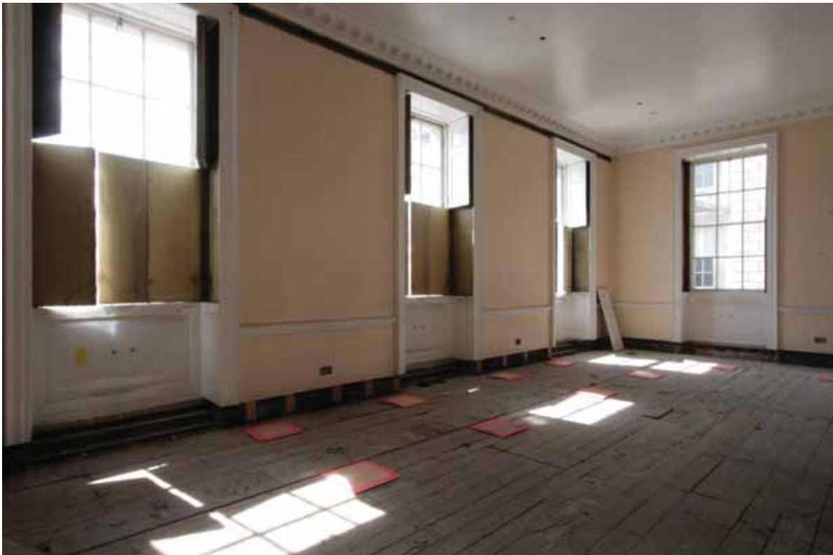
Plate 482: West (left) and north (right) walls in Room F09, looking north-west (EAF10 241)
