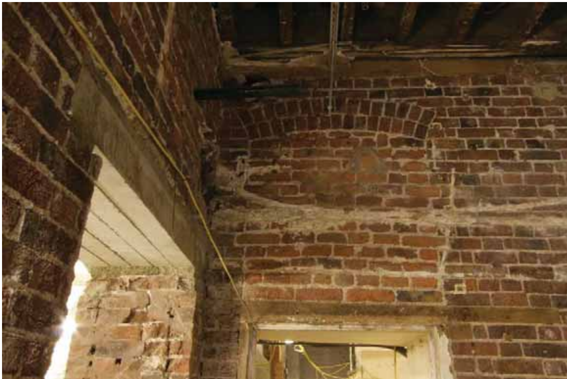
Plate 107b: North (left) and east (right) walls of Room B62, looking north-east; the doorway in the north wall was inserted in 2011 (EAF10 A-D101 001)
