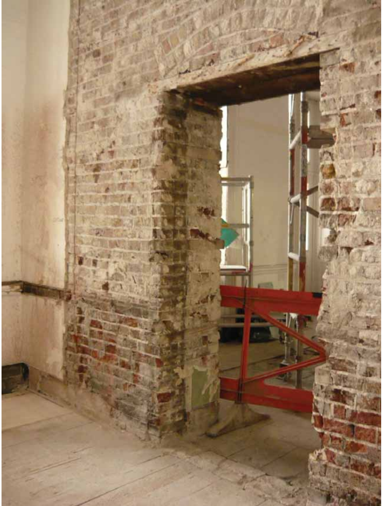
Plate 341: Doorway in the centre of the north wall in Room G41, looking north-west (EAF10 BHD8 (63))
