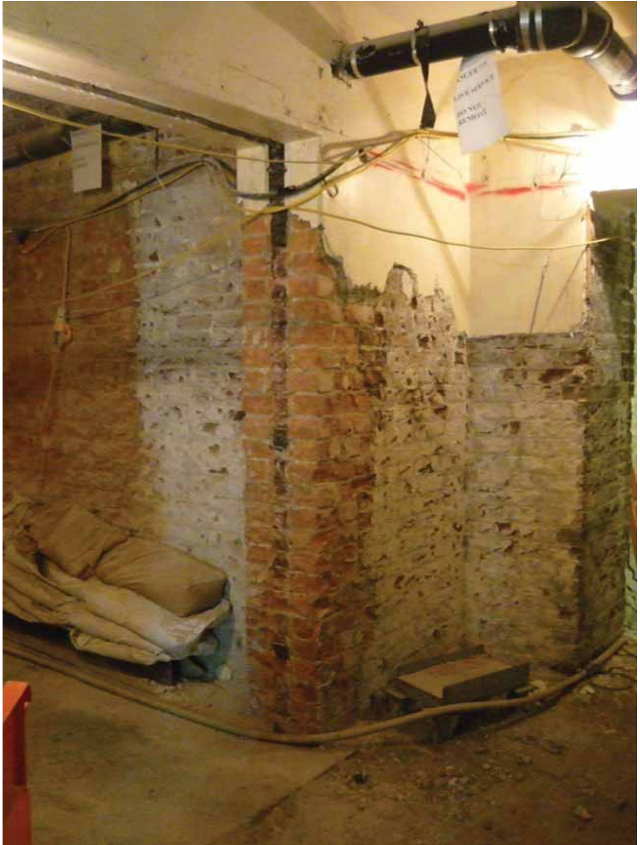
Plate 87a: View north-east from Corridor 1D (right) to Corridor 1C (left) (EAF10 BDH6(66))
