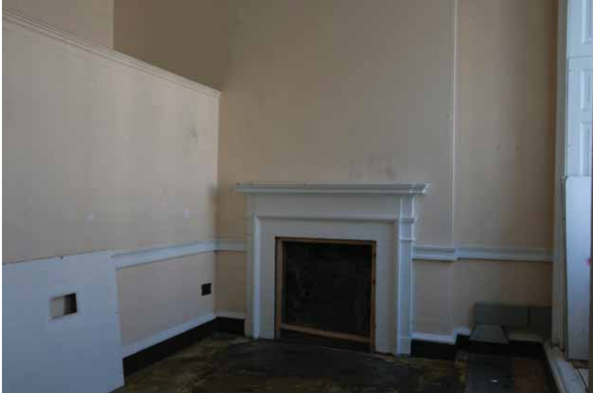
Plate 545: Fireplace (type 6) in the north wall of Room F27, looking north (EAF10 153)
