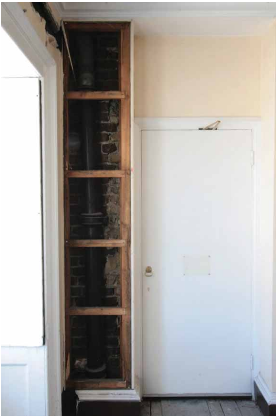
Plate 575: Boxed in pipe in the north-west corner of Room S09, looking north (EAF10 222)
