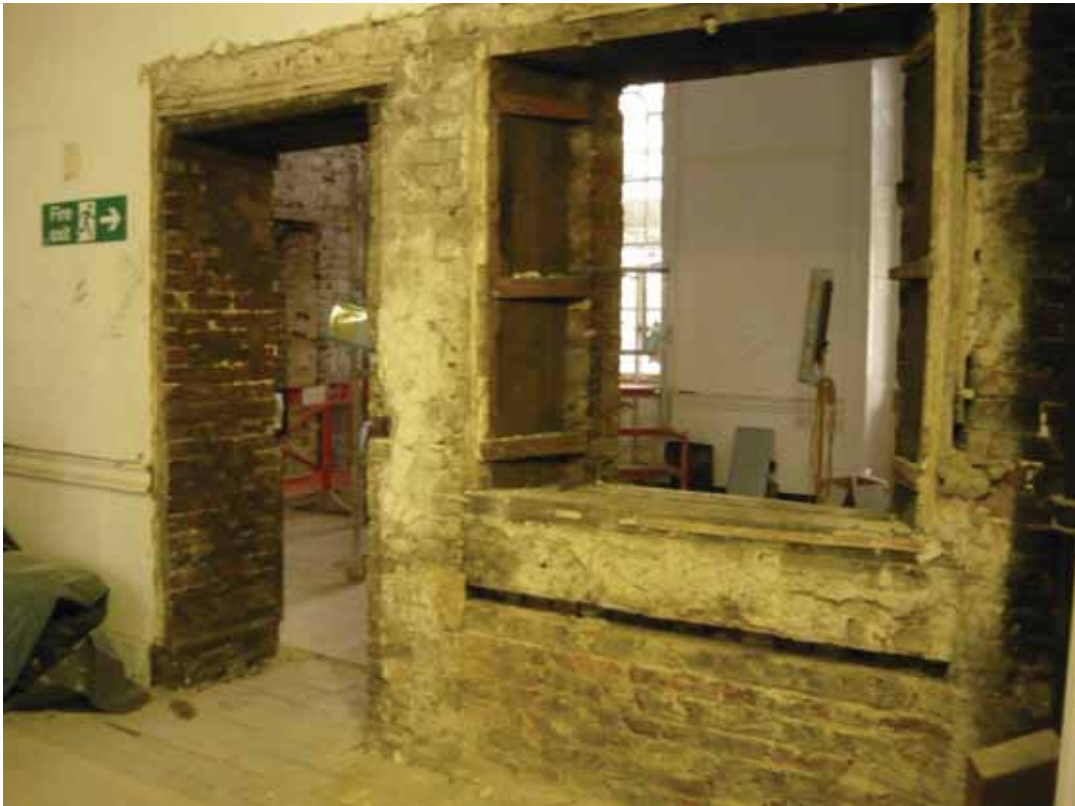
Plate 389: Removal of plaster from the west wall of Corridor 07G looking south-west (EAF10 BHD8 (66))
