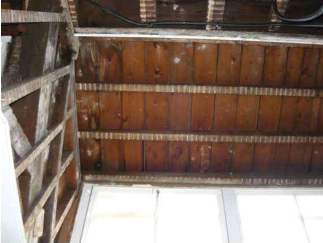
Plate 698: Dormer in the east side of the roof in Room T09, looking east (EAF10 BHD10 (78))
