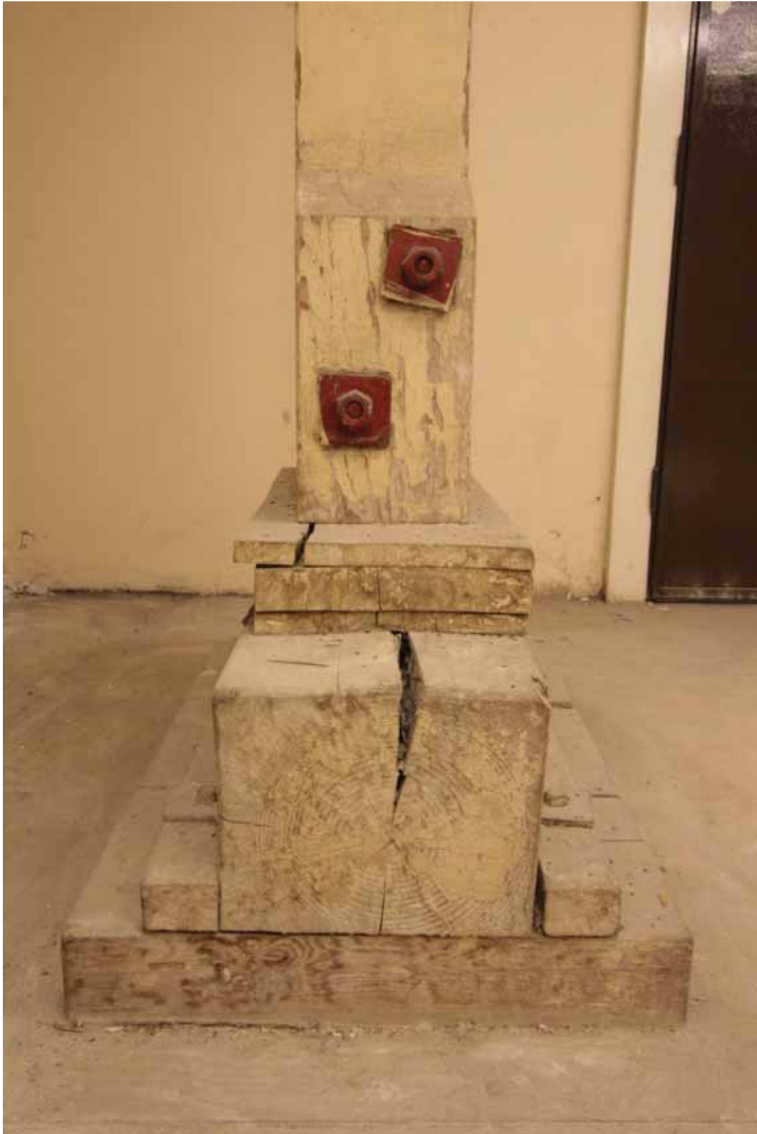
Plate 57: World War Two shoring base in the north-east corner of Room B48A, looking east (EAF10 D100 037)
