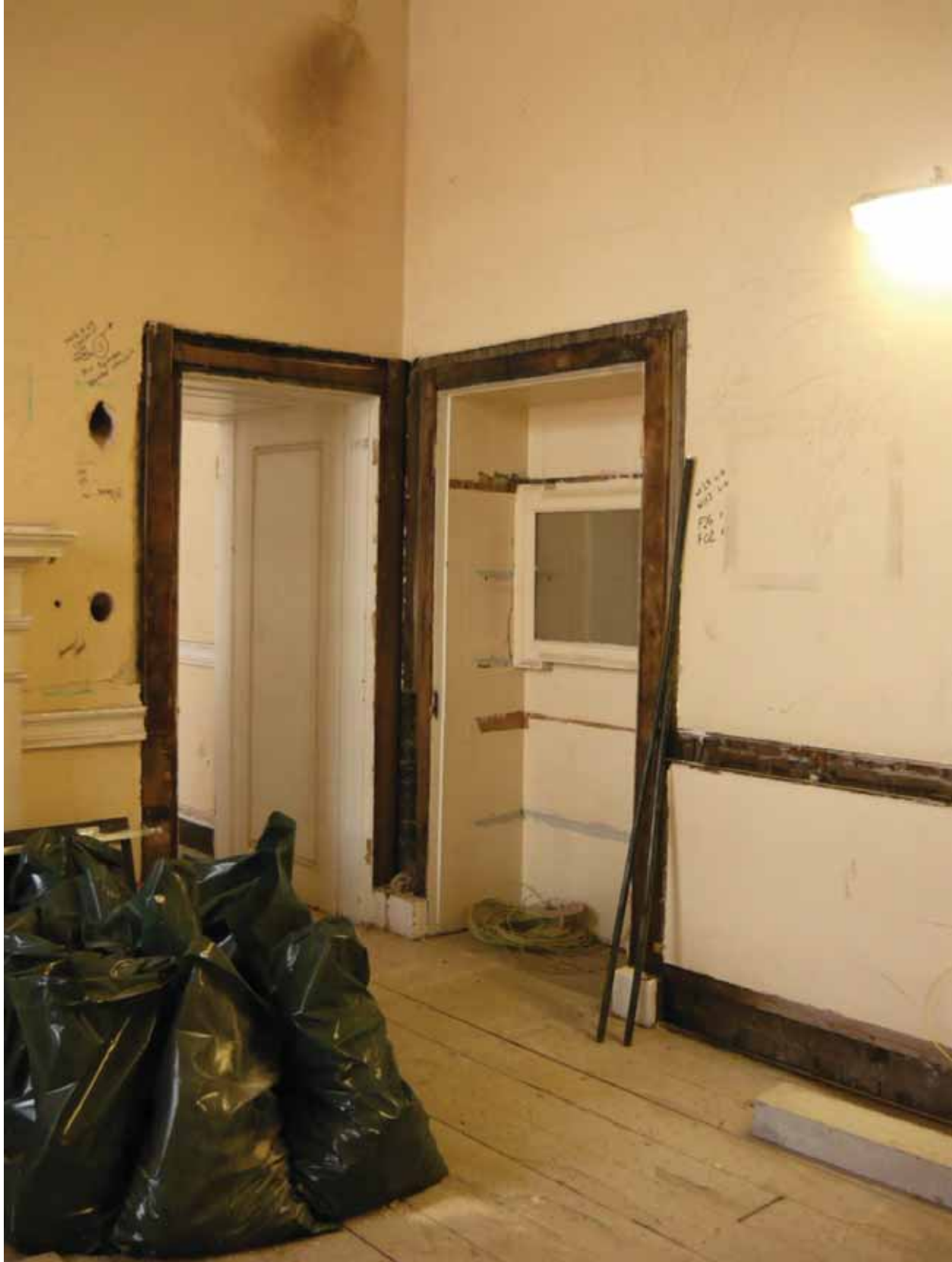
Plate 480: North (left) and east (right) walls in Room F05, looking north-east (EAF10 BHD8 (10))
