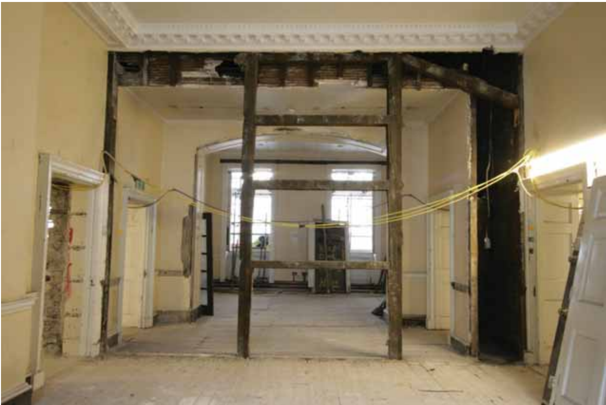
Plate 519: Remains of west partition wall in Room F16, looking west (EAF10 A100 020)
