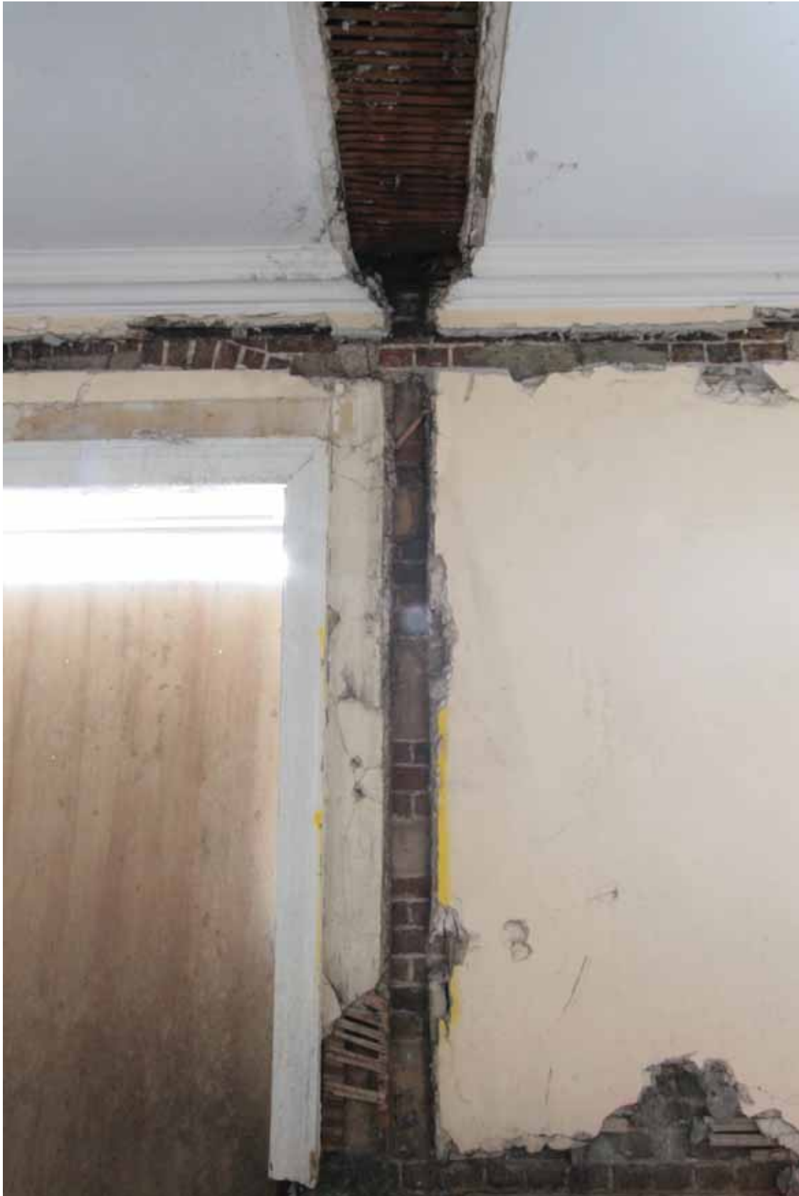
Plate 566: Scar of removed partition wall in the west wall of Room S02/S03, looking west (EAF10 229)
