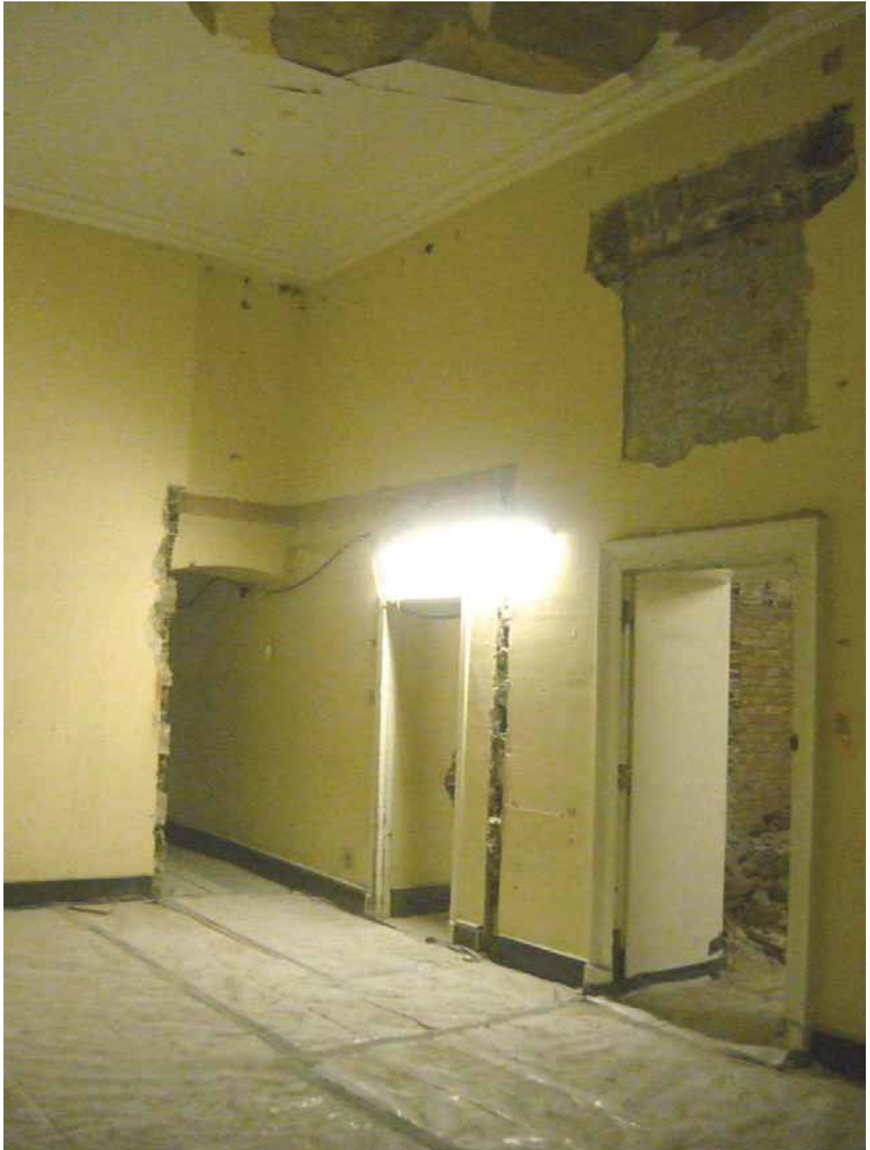
Plate 278: South (left) and west (right) walls in Room M23, looking south-west (EAF10 BHD6 (71))
