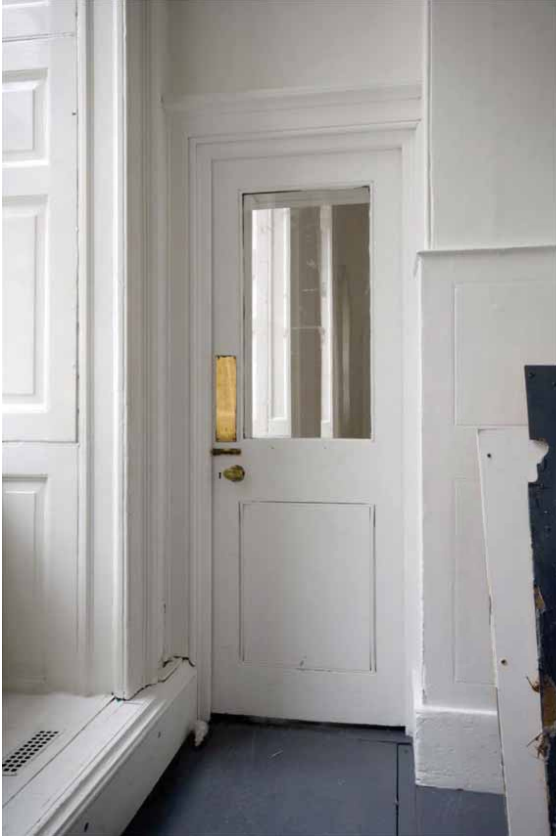
Plate 405: Doorway (type 42) in the south wall of Room G40, looking south (DSC_0822 sitecode EAF10 © PCA Ltd 2010)
