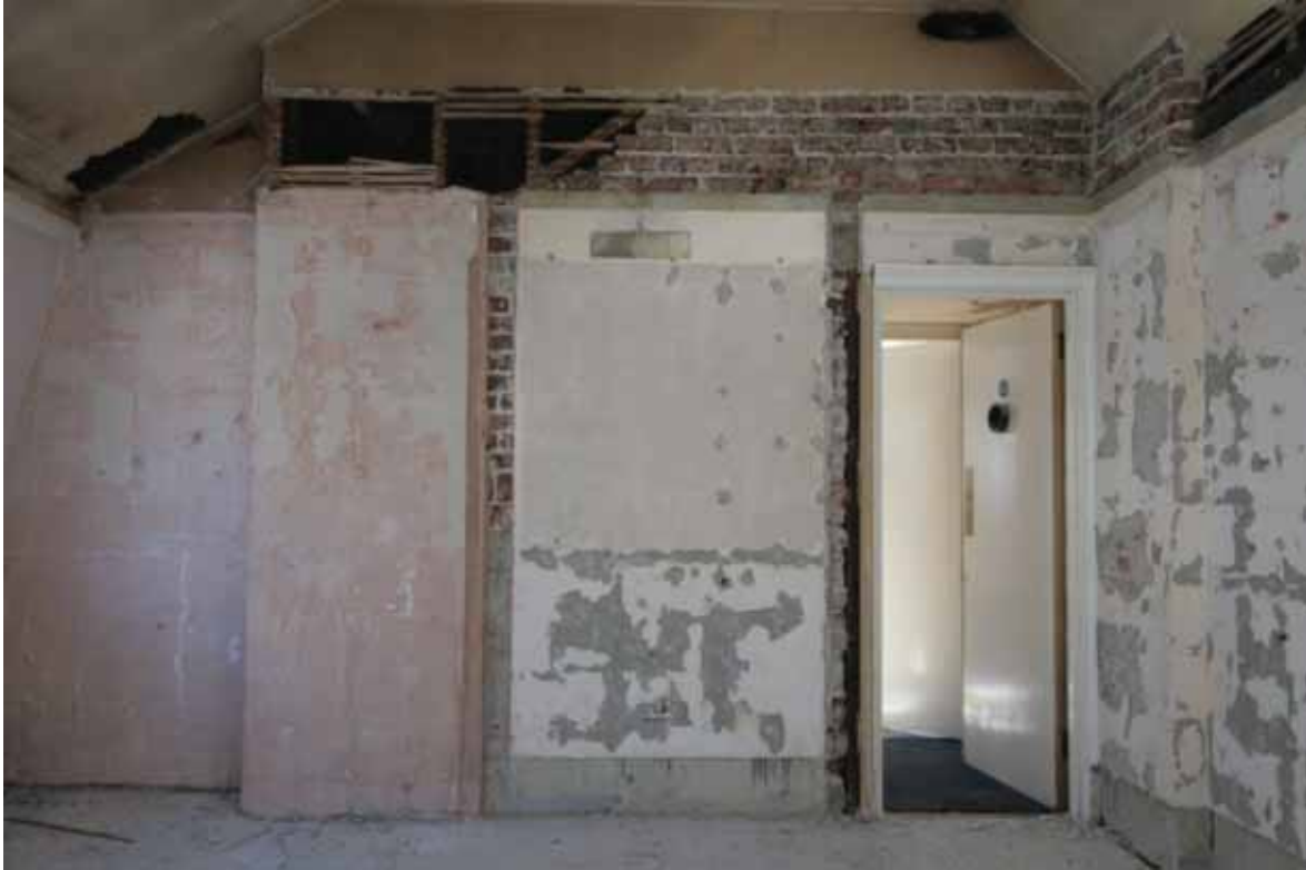
Plate 761: South (left and centre) and west (right) walls in Room T20, looking south (EAF10 196a)
