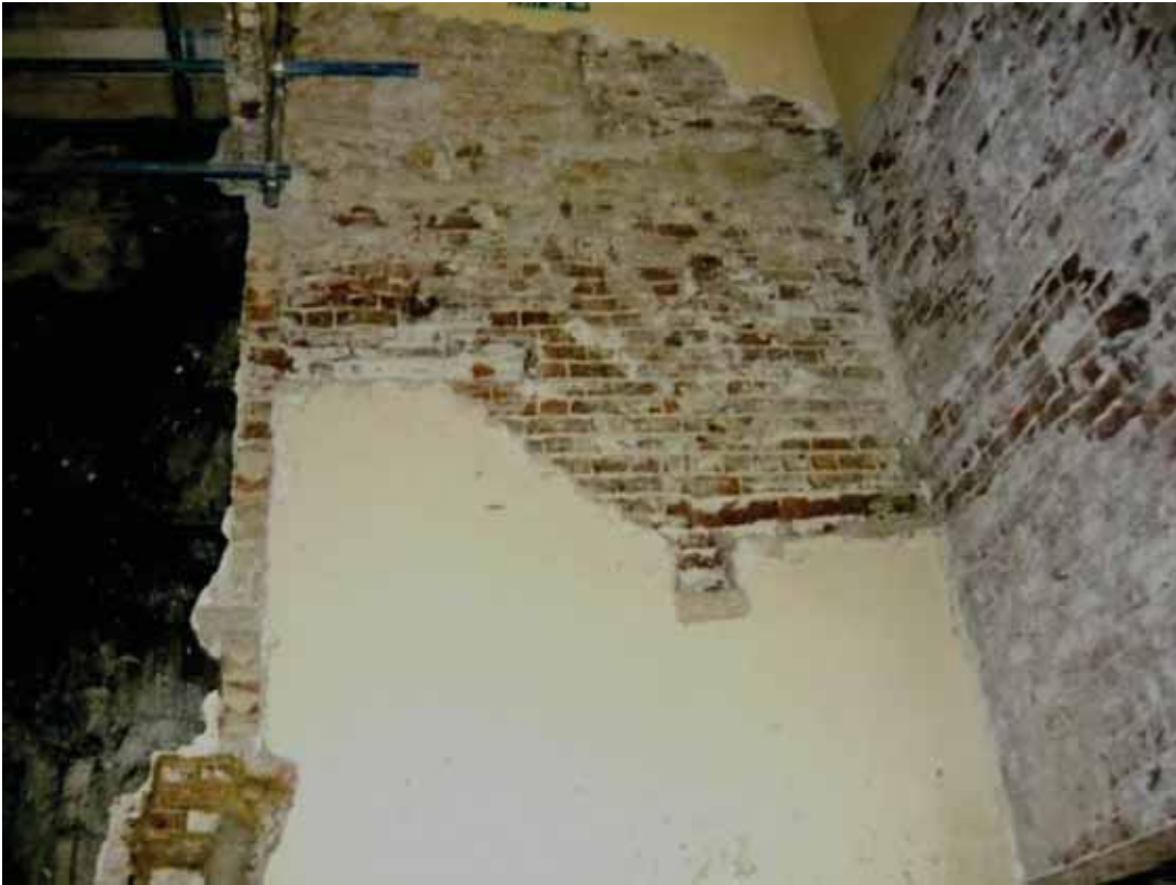
Plate 258: West (left and centre) and north (right) walls (upper level) of Corridor 06LG looking north-west (EAF10 BHD8 (106))
