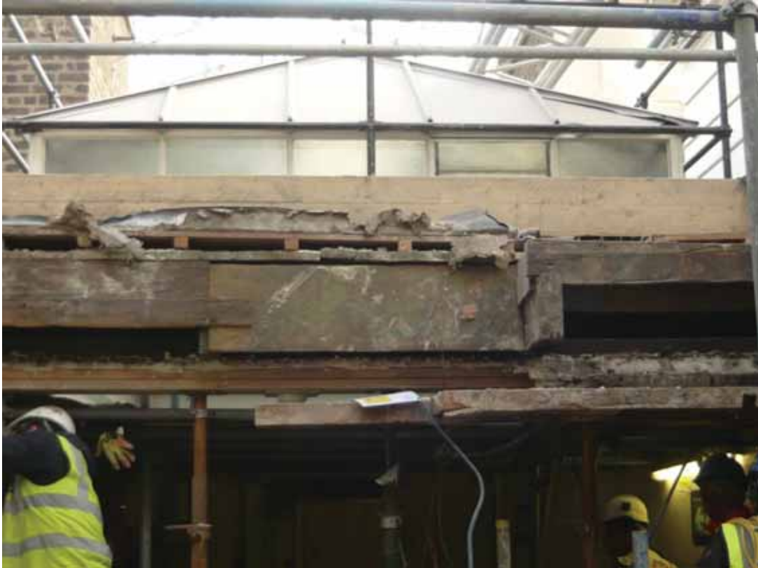
Plate 810: Lantern skylight over Corridor 05T and removed south wall of Cupboard 01T and Corridor 04T, looking south (EAF10 BHD8 (53))
