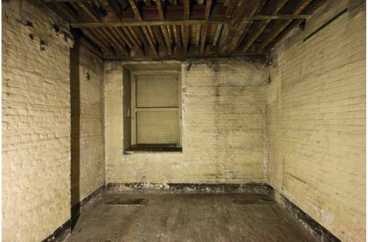
Plate 140: East wall of Room B51, looking east (DSC_1438 _sitecode EAF10_© PCA Ltd 2010)
