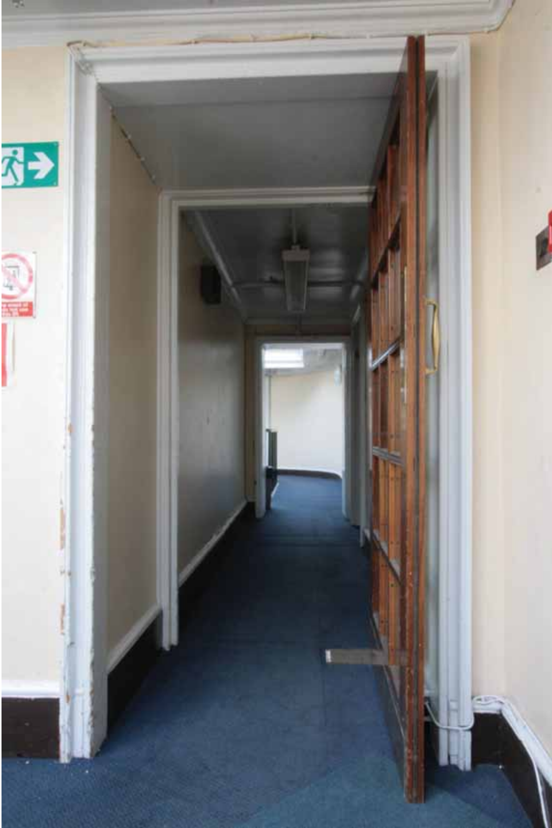
Plate 712: Doorway at the west side of the south wall in Corridor 03T looking south through Corridor 04T to Corridor 05T beyond (EAF10 36)
