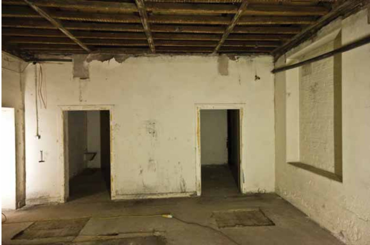
Plate 30: Doorways in the south wall of Rooms B47A, looking south (DSC_1449 _sitecode EAF10_© PCA Ltd 2010 )
