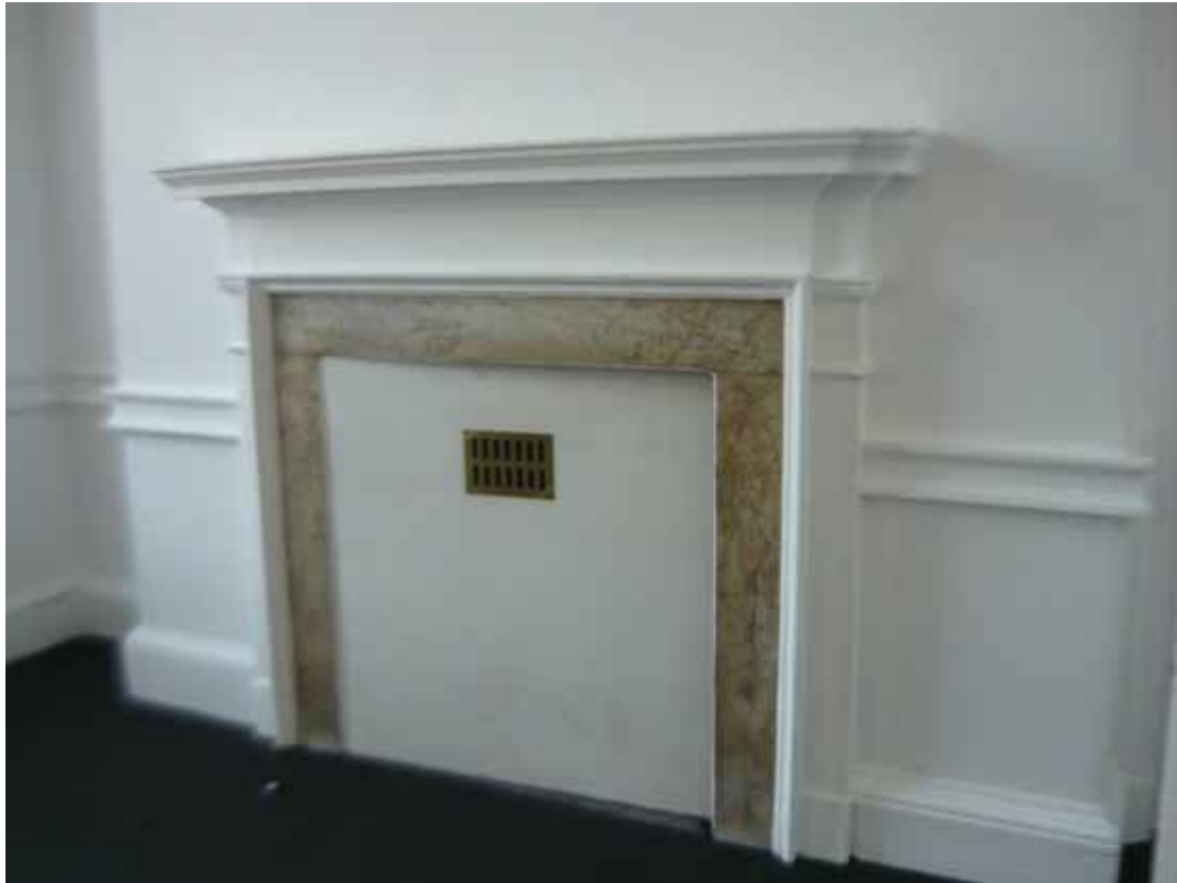
Plate 352: Fireplace (type 6) in the north wall of Room G02, looking north-west (EAF10 BHD1 (51))
