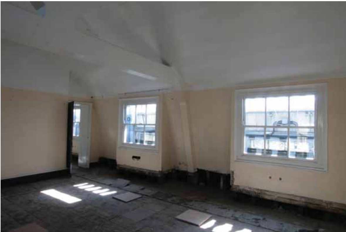
Plate 658: South (left) and west (right) walls in Room T119, looking south-west (EAF10 205)
