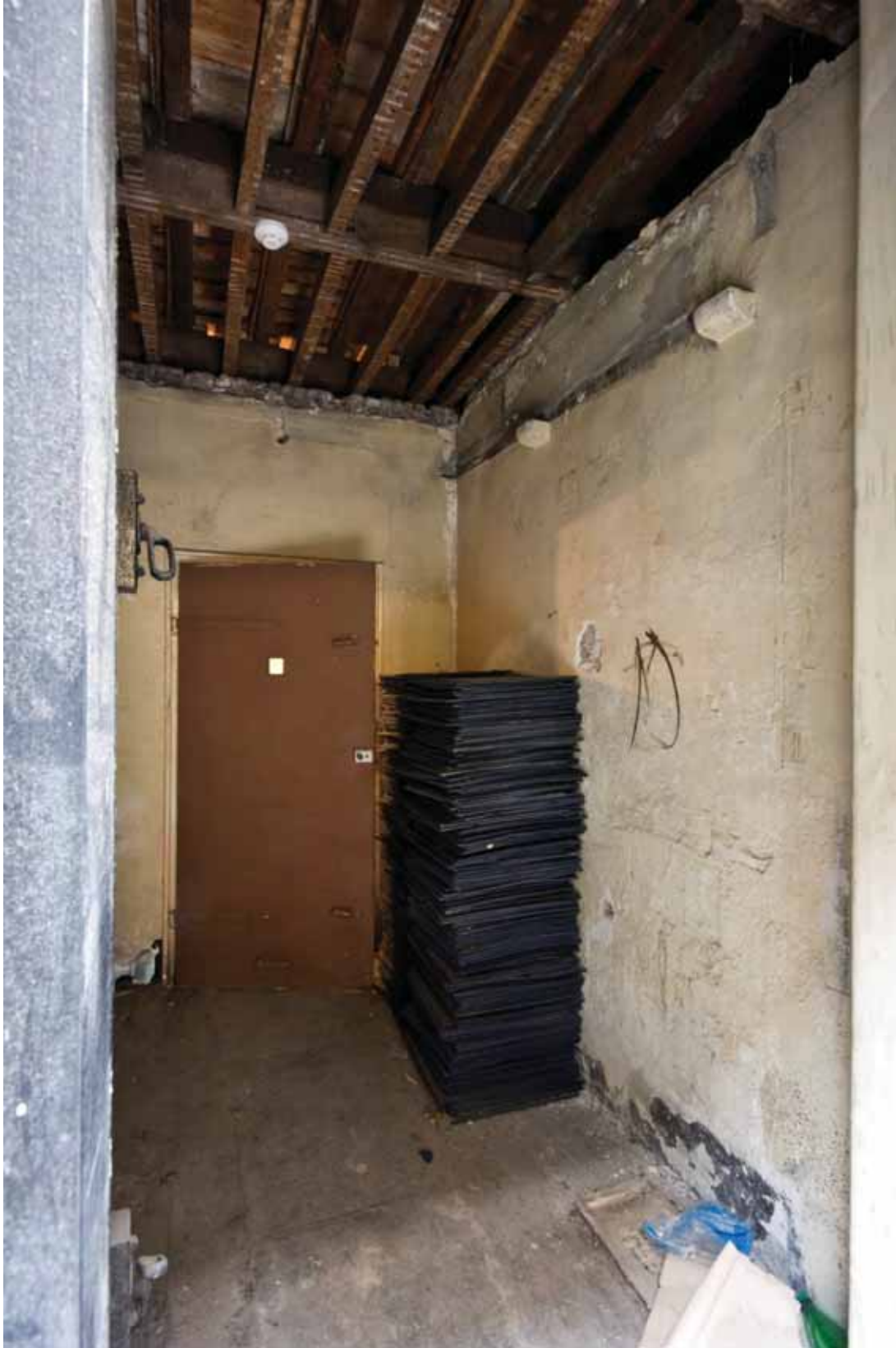
Plate 157: Doorway in the west wall of Room B54B, looking west (DSC_1508 _sitecode EAF10_© PCA Ltd 2010 _1)
