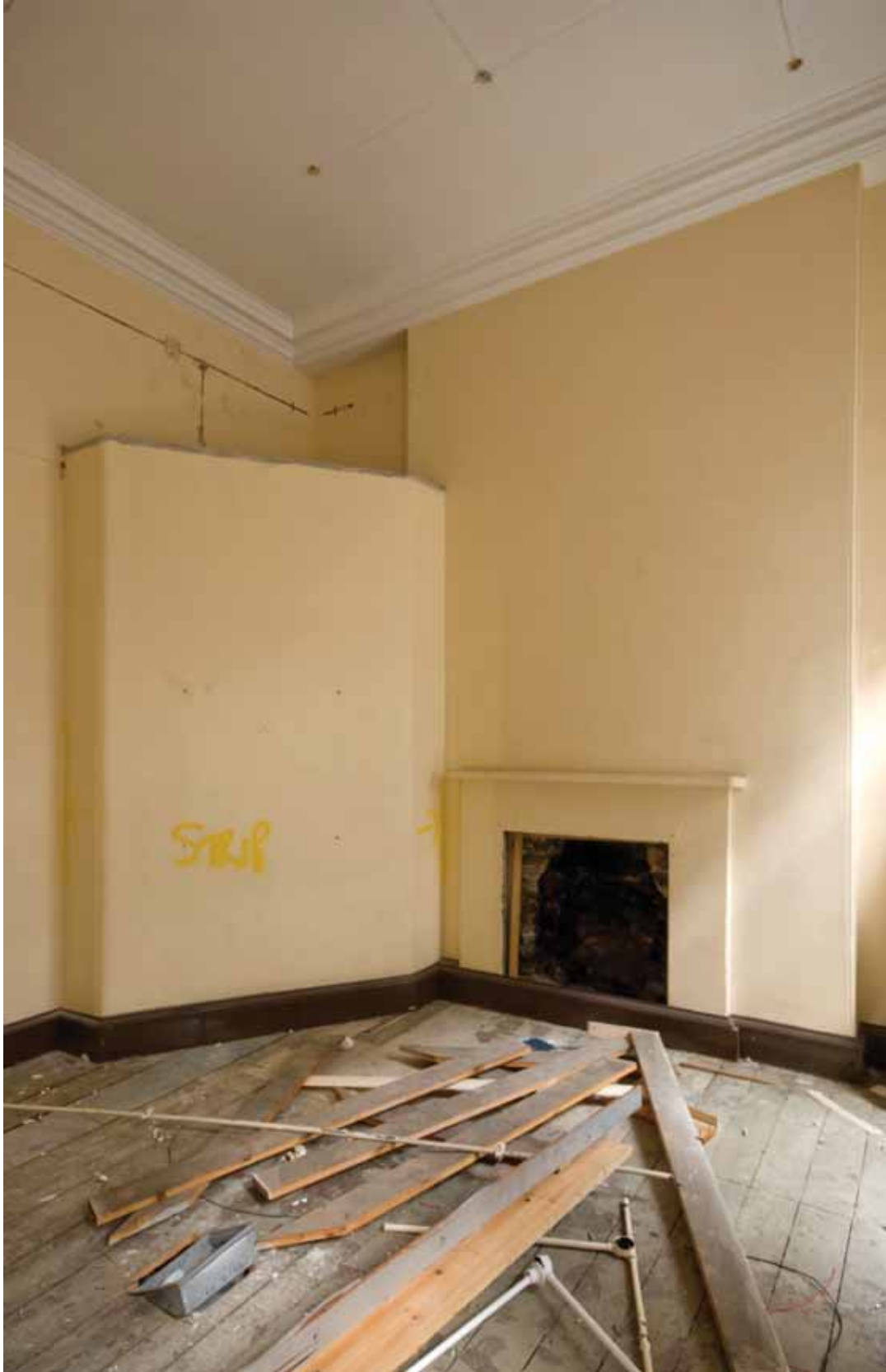
Plate 317: West (left) and north (right) walls in Room M29a, looking north-west (EAF10 LG100 0975)
