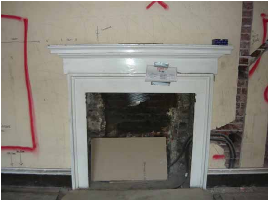
Plate 552: Fireplace (type 4) at the north end of the east wall in Room S96, looking east (EAF10 BHD12 (5))
