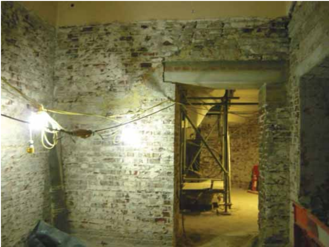
Plate 106: North wall of Corridor 7 (concrete lintel is a 2011 replacement), looking north (EAF10 BHD13 (16))
