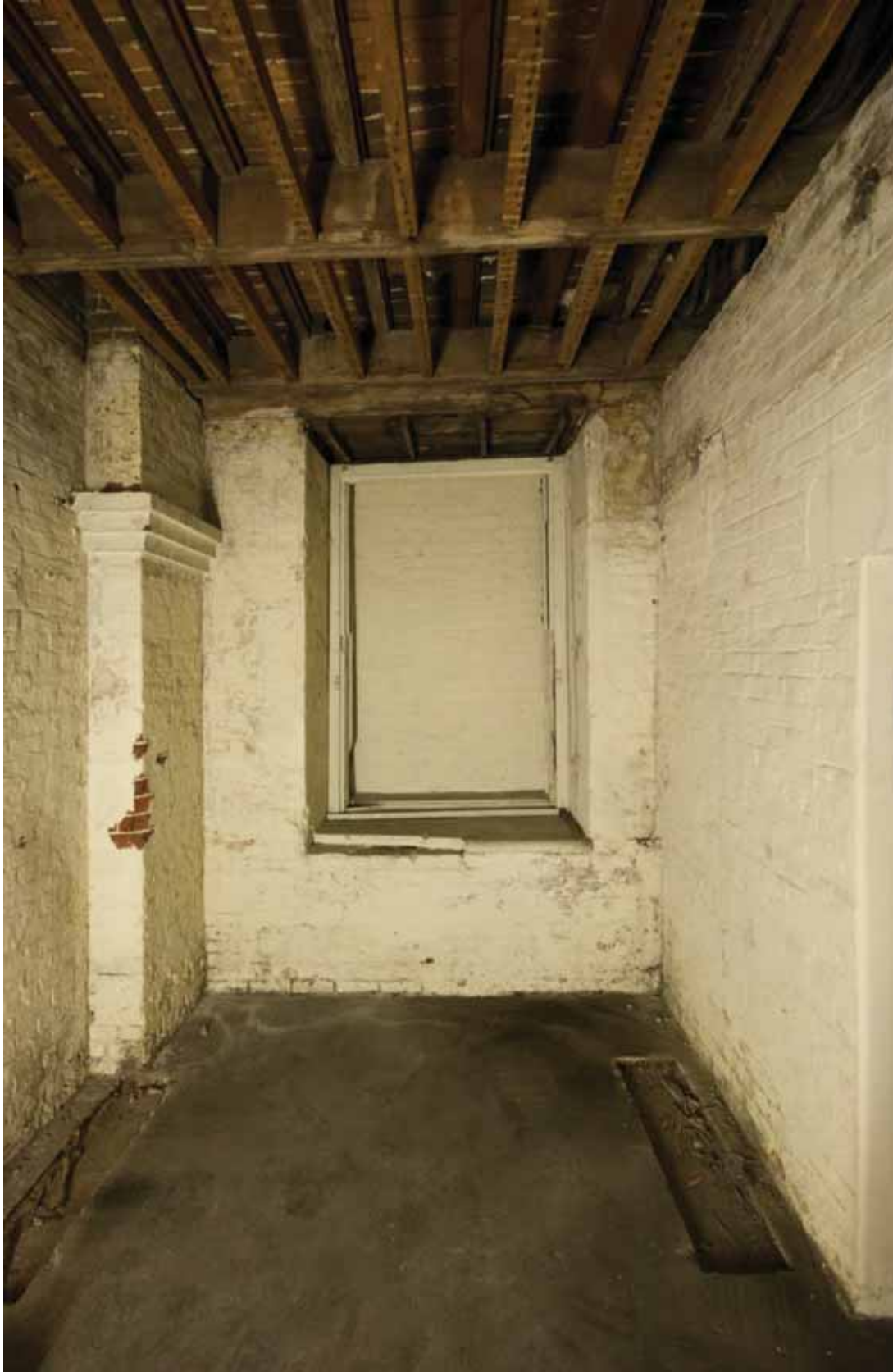
Plate 112: East wall of Room B49A, looking east (DSC_1405 _sitecode EAF10_© PCA Ltd 2010)
