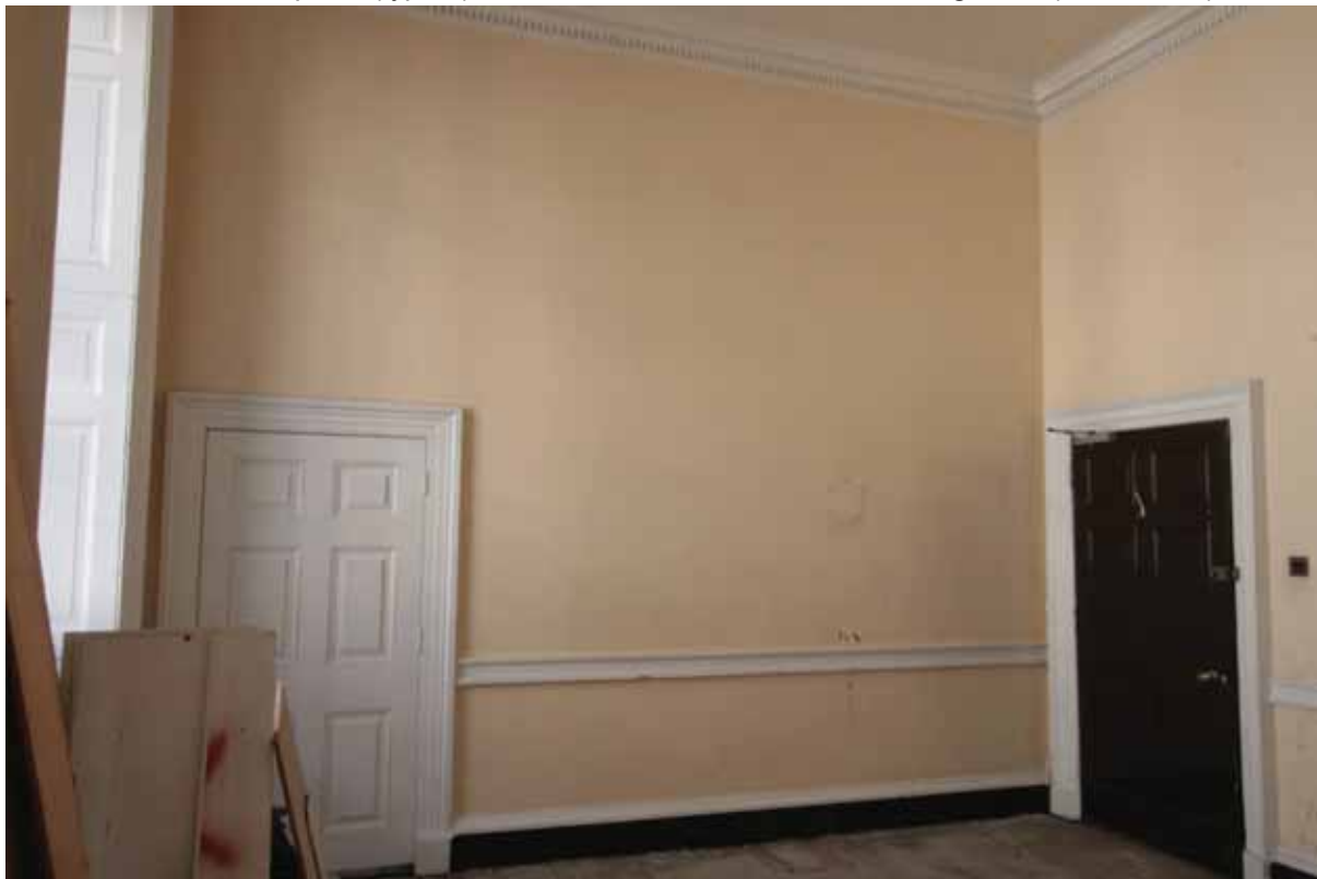
Plate 531: East (far left), south (centre) and west (right) walls in Room F18, looking south (EAF10 179)
