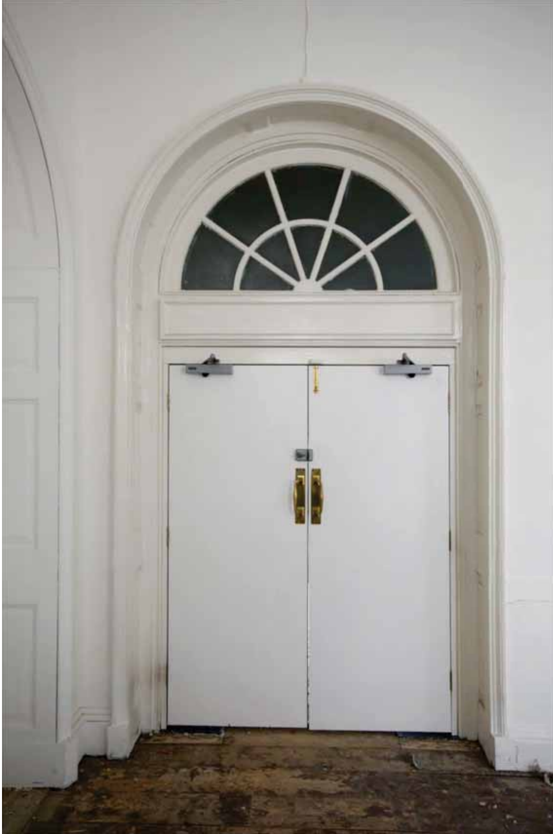
Plate 404: Doorway (type 43) at the south end of the west wall of Room G39, looking west (DSC_0820 sitecode EAF10 © PCA Ltd 2010)
