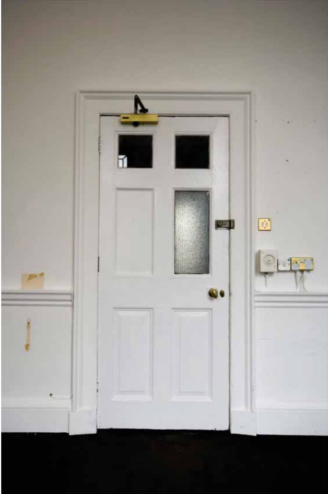
Plate 346: Doorway (type 41) in the east wall of Room G01, looking east (DSC_0835 sitecode EAF10 © PCA Ltd 2010)
