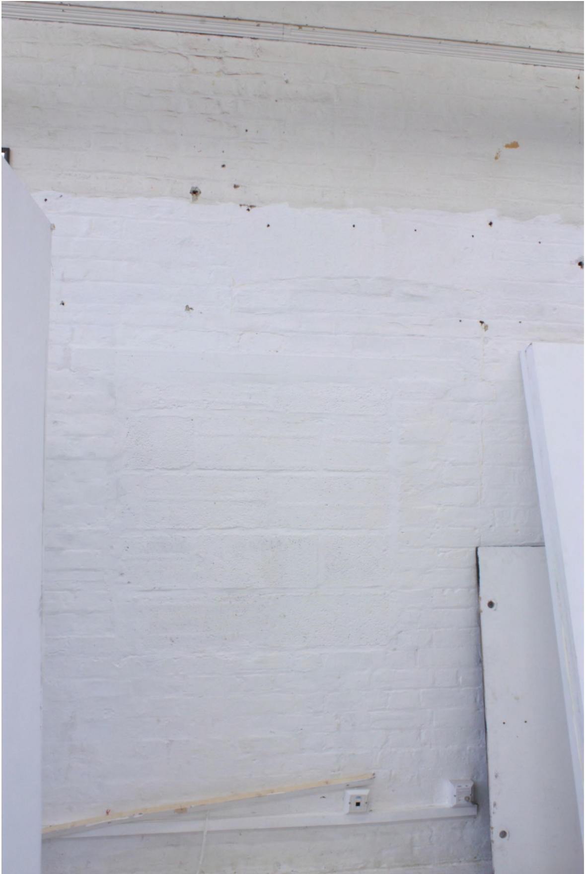
Plate 17b: Former doorway converted to a window which was then blocked in the east wall of Room 6 in Block 200, looking east (D4/13)
