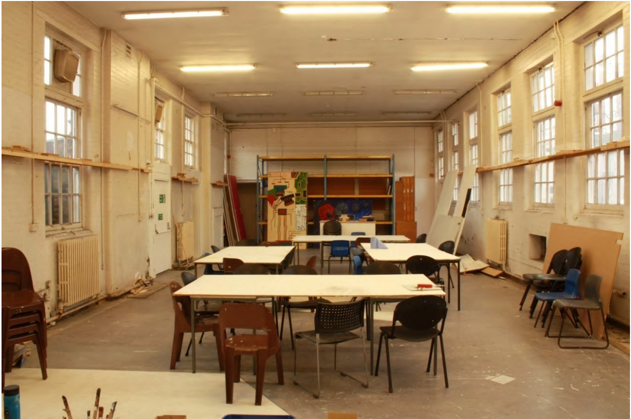
Plate 16: South (left), west (centre) and north (right) walls of Room 6 in Block 200, looking west (D4/19)
