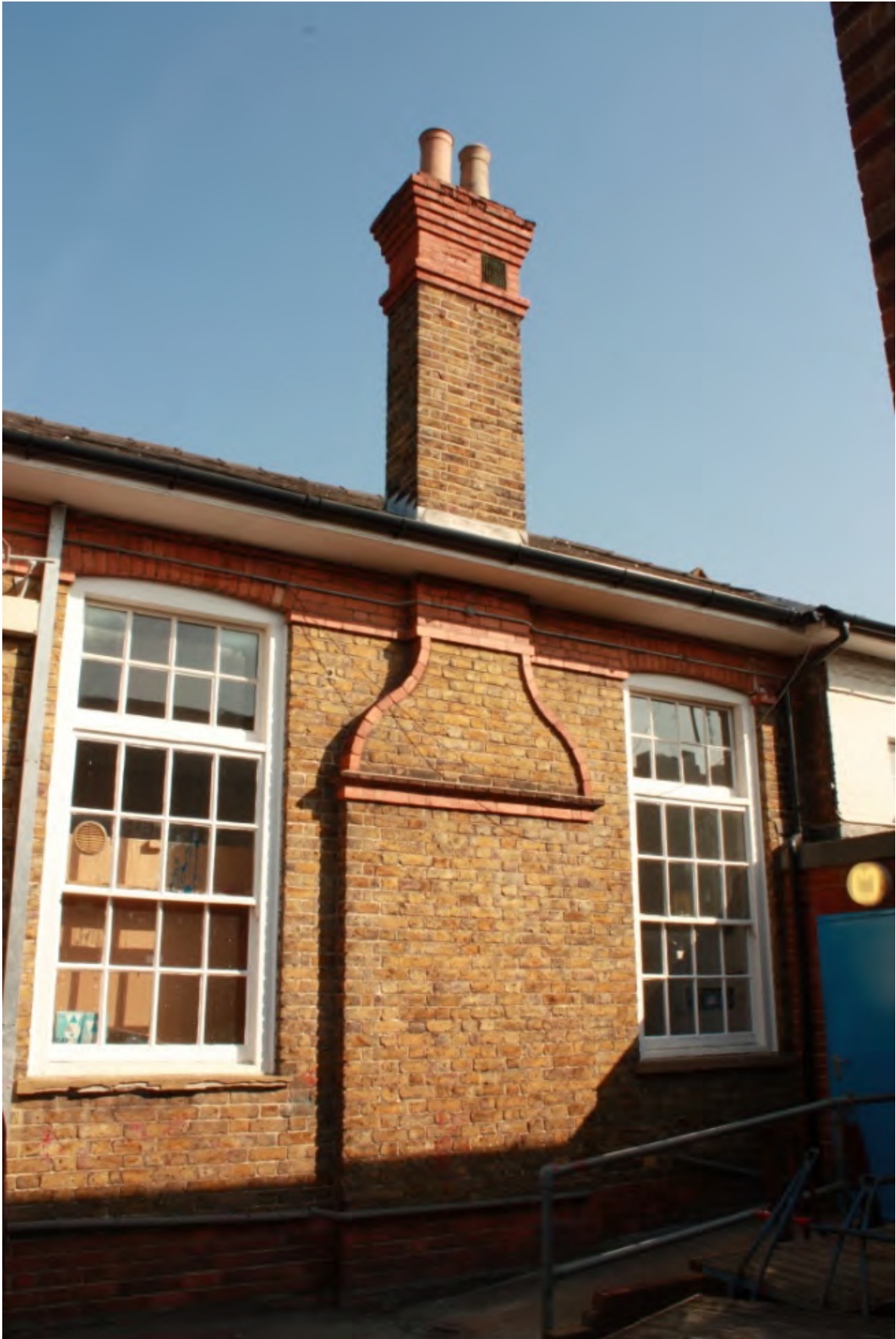
Plate 6: Chimney breast and stack on the south elevation of Block 200, looking north-east (D1/24)
