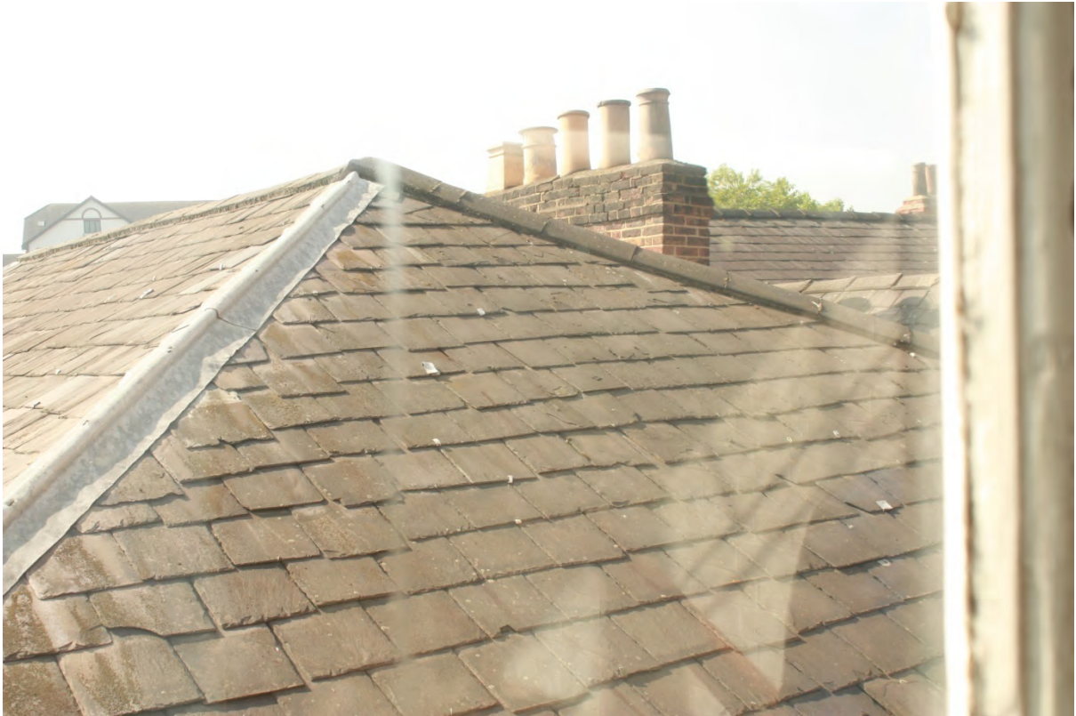
Plate 4g: Hipped roof over Room 1 of the Penny Gallery, looking south-west (D2/3)
