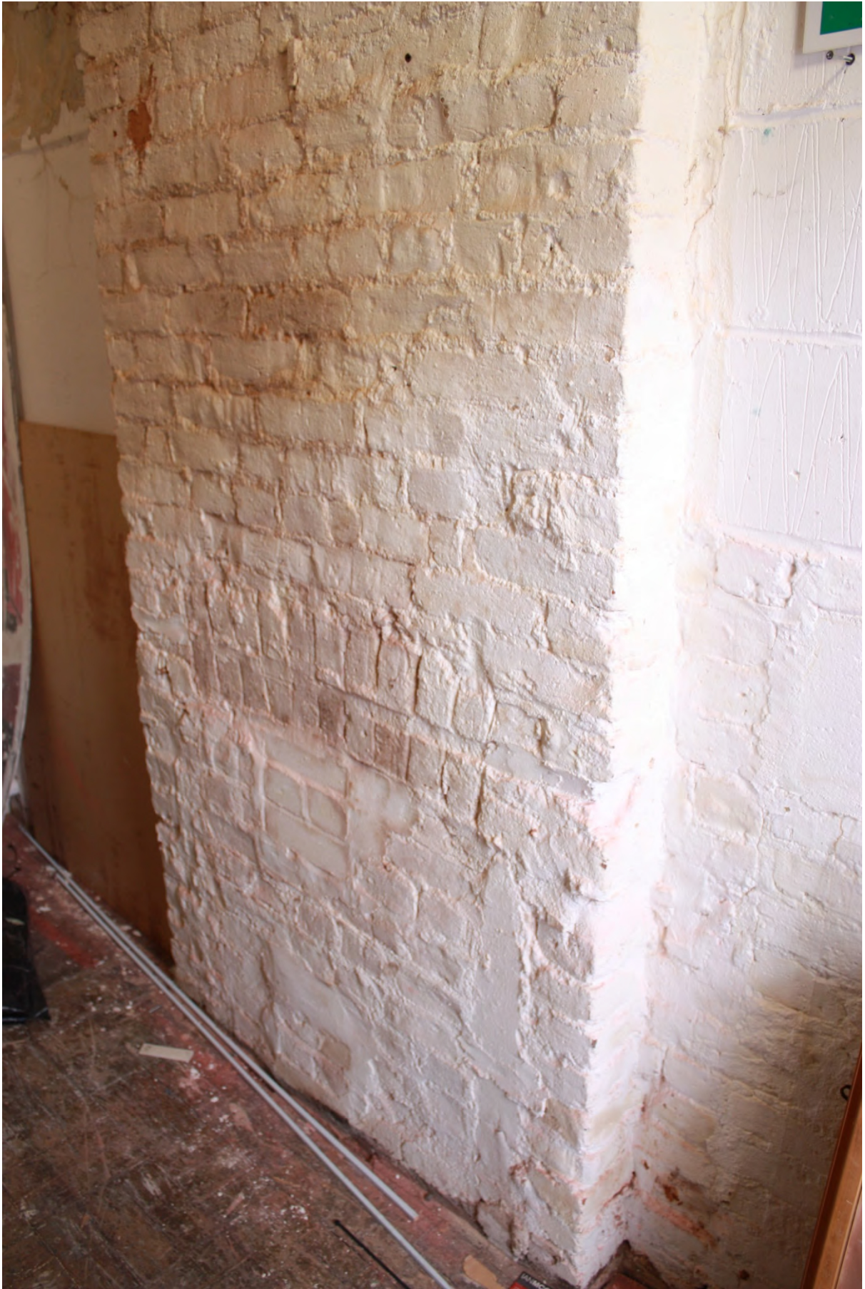
Plate 14a: Blocked fireplace in the east wall of Room 3, looking north-east (D2/27)
