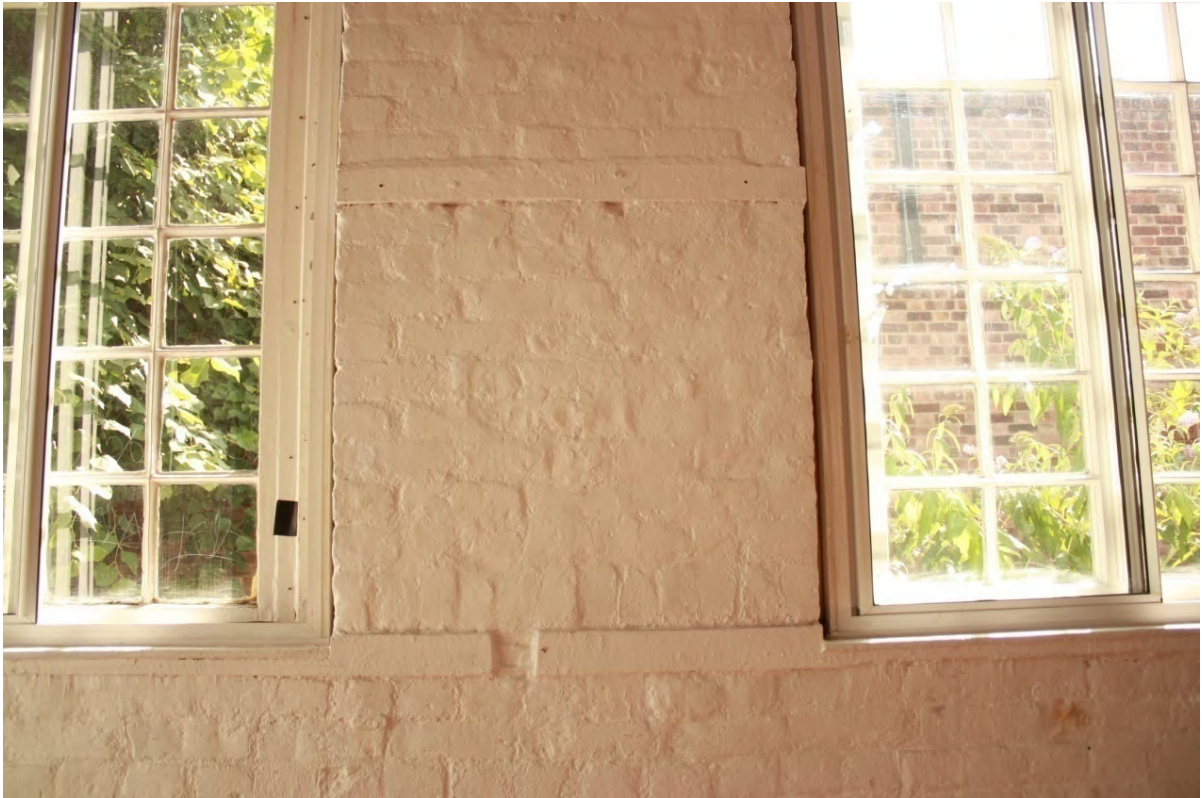
Plate 13: South internal wall of Room 1 in the Penny Gallery showing timber battens embedded in the brickwork, looking south (D2/23)
