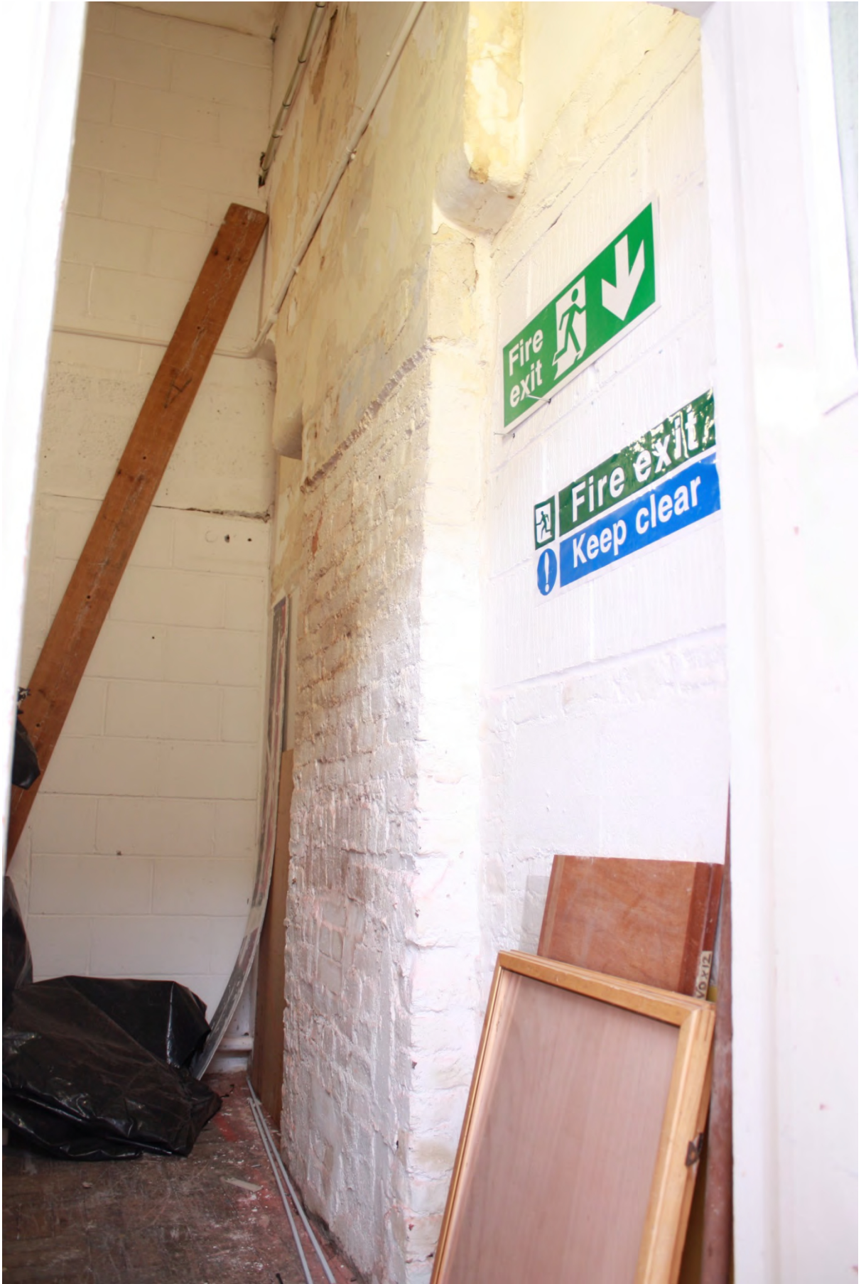
Plate 14b: Blocked fireplace in the east wall of Room 3, looking north-east (D2/27)
