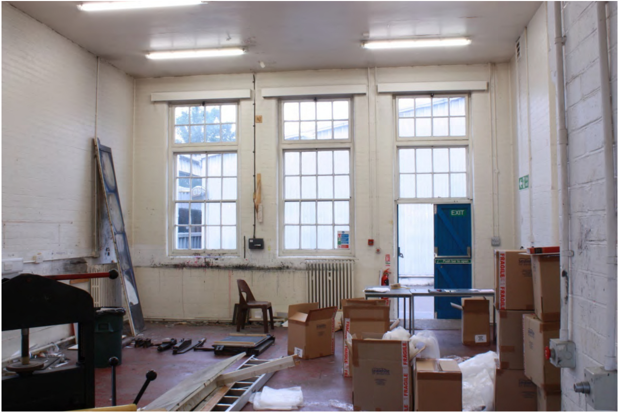
Plate 19: West (left), north (centre) and east (right) walls of Room 10a in Block 200, looking north (D3/30)
