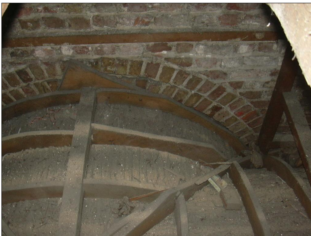
Figure 12: Floor void above the East Court South range, second floor corridor (Room 227), revealing the timber vaulting for double-height ground floor corridor (↑E)
