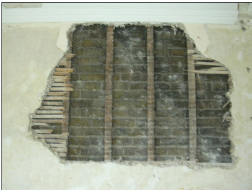
Figure 11: Room 214, differential staining on east (external) wall
