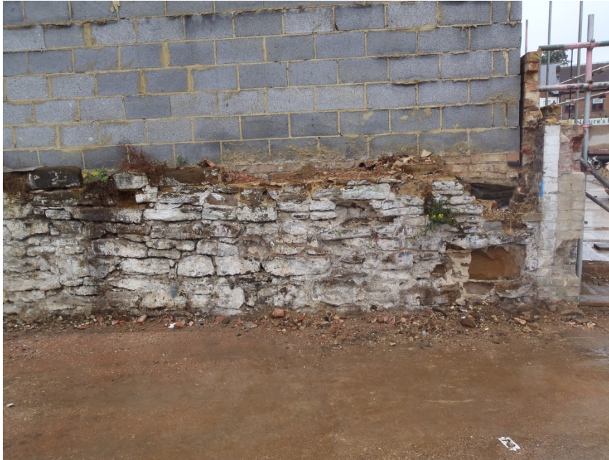
Plate 11: Old sandstone wall used as foundation for Maple Mews property. The wall shares its alignment with the north-south ditches of Saxo-Norman/early medieval date suggesting a continuation of alignments
