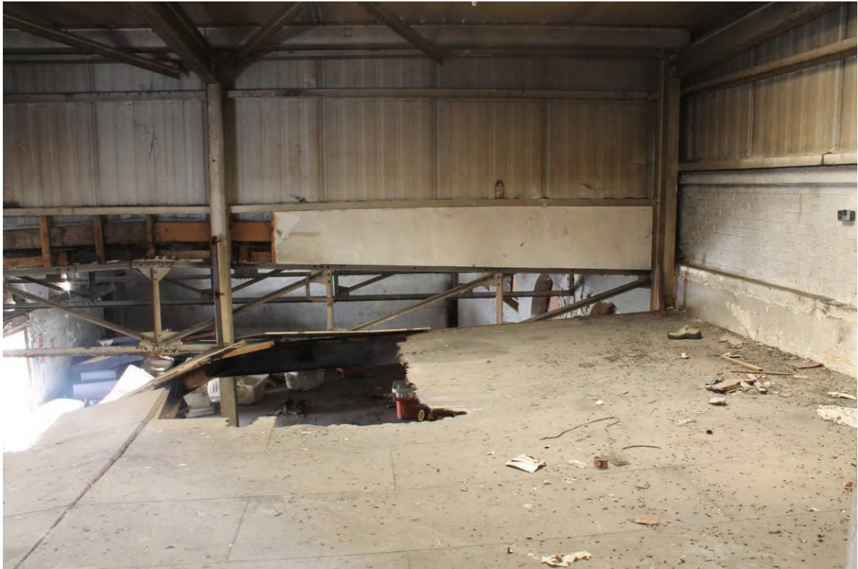
Plate 35 Mezzanine floor in Tidal Basin Road Post and Sorting Office, looking south
