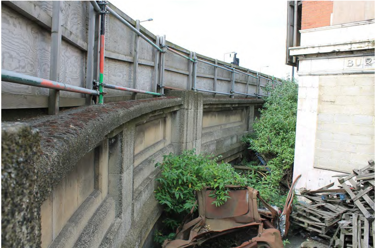
Plate 5 Access ramp to Silvertown Flyover (left) with Tidal Basin Tavern (right), looking west
