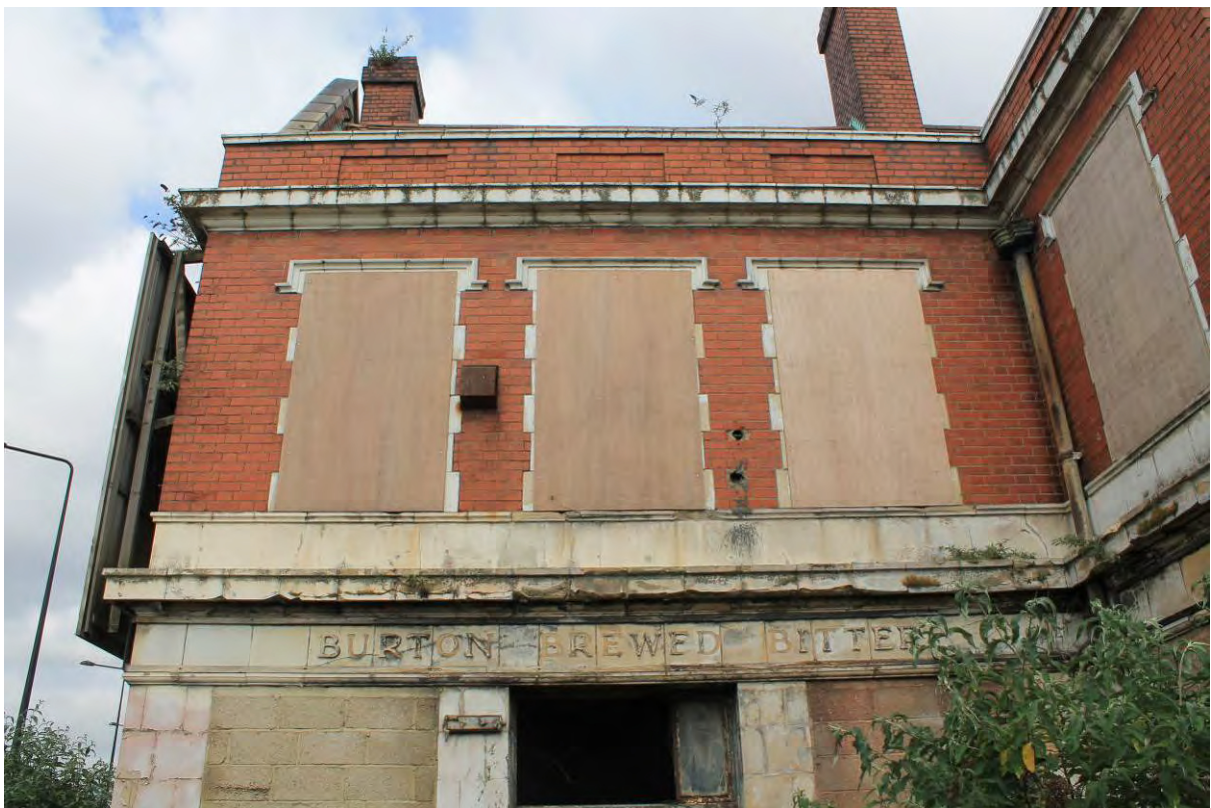
Plate 4 Tidal Basin Tavern south end of the east elevation at first floor level, looking west
