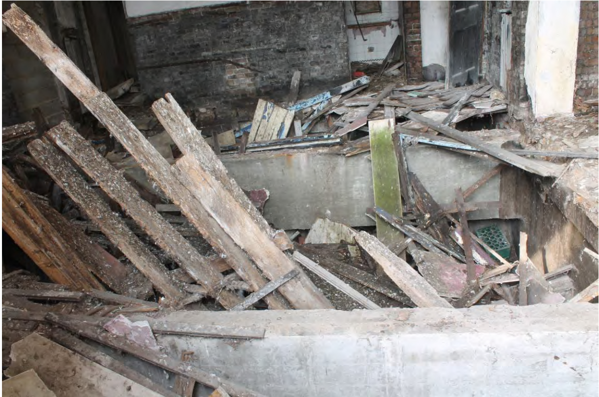
Plate 43 Concrete bridging beams over basement storey in the southern part of the front (eastern) bar of Tidal Basin Tavern, looking west
