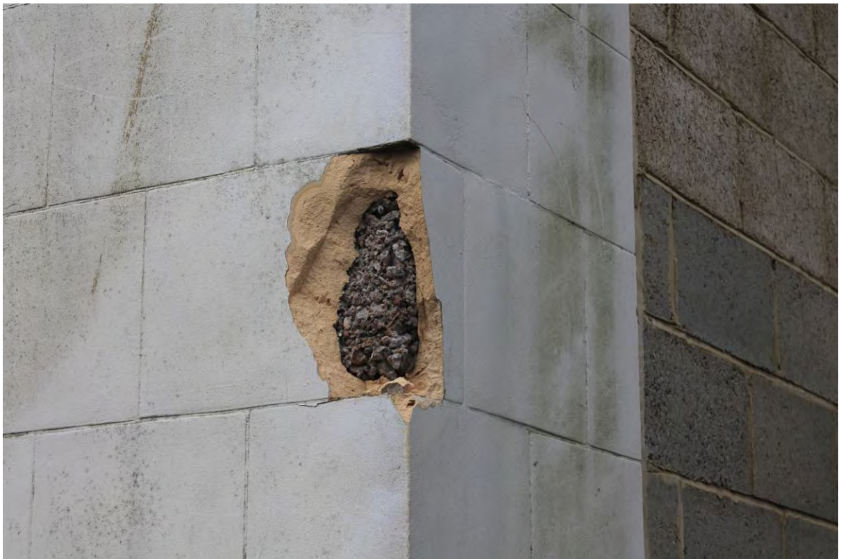
Plate 44 Concrete filled cavity within terracotta wall tiles at the south-east corner of the Tidal Basin Tavern, looking north-west
