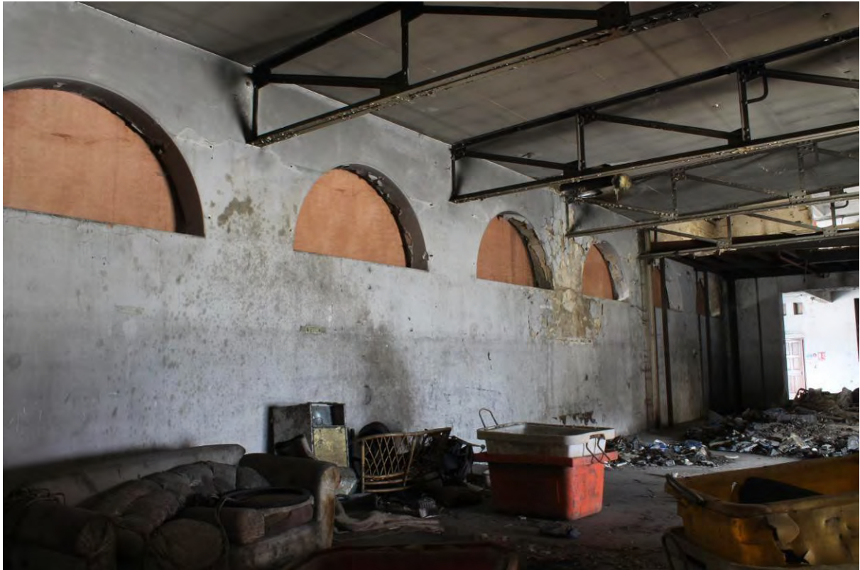
Plate 23 Western wall showing half round windows in GF7 of Tidal Basin Road Post and Sorting Office, looking north-west
