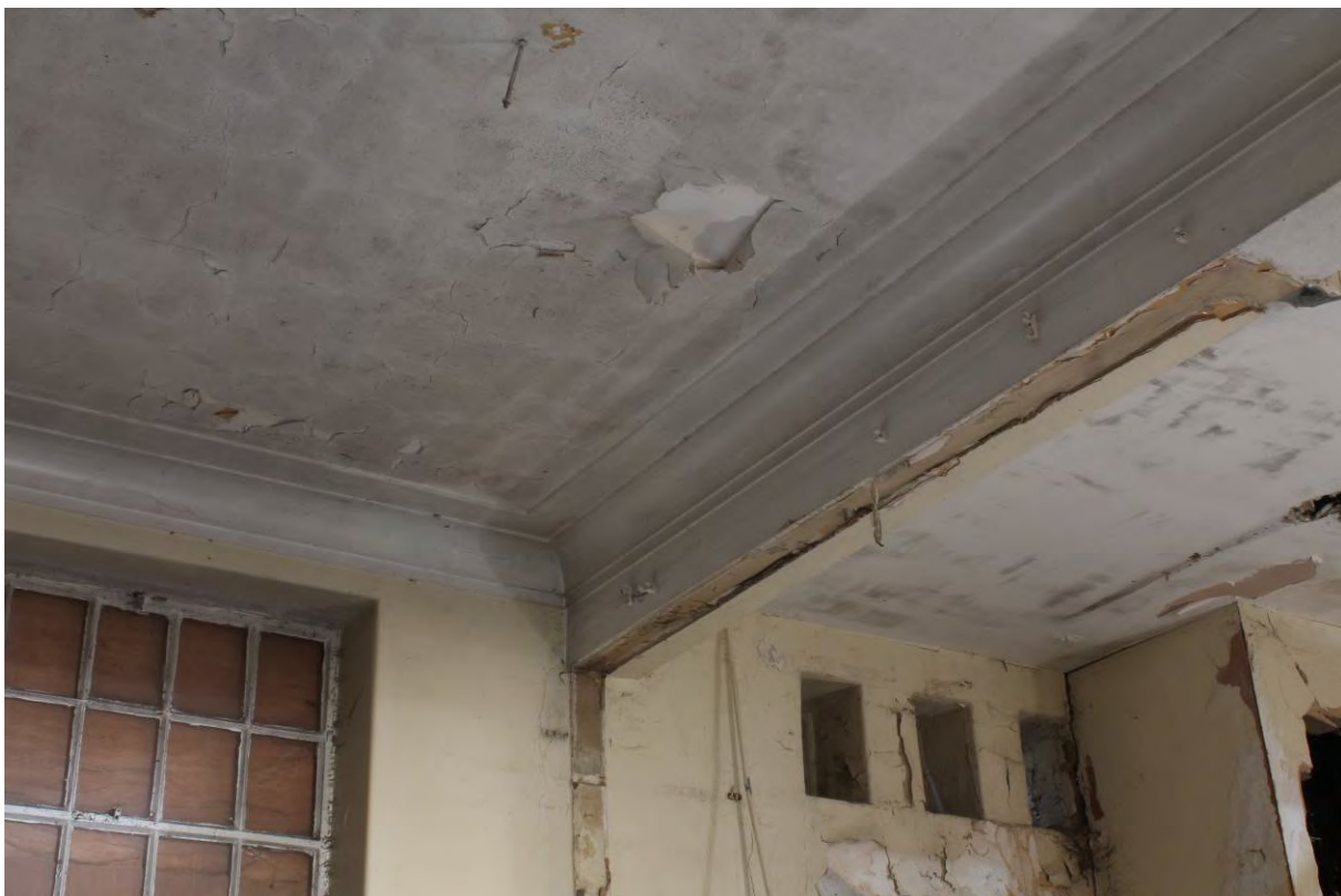
Plate 28 Ceiling cornice and downstand in GF2 in Tidal Basin Road Post and Sorting Office, looking north-east towards the north wall
