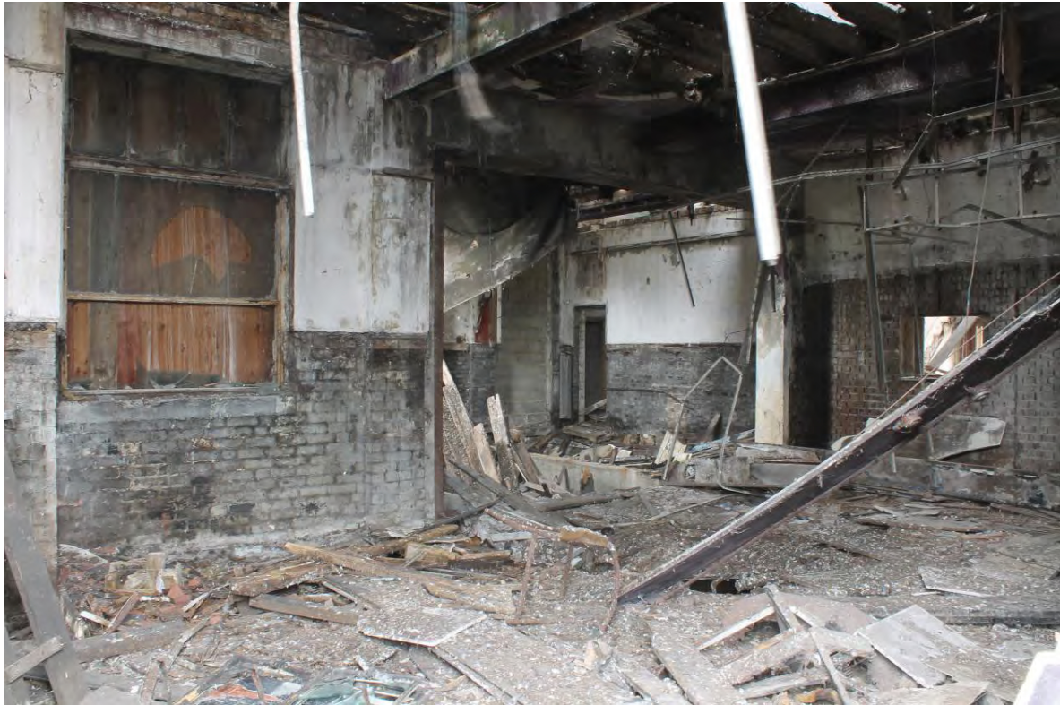
Plate 39 Central and southern part of the front (eastern) bar of Tidal Basin Tavern, looking south-west
