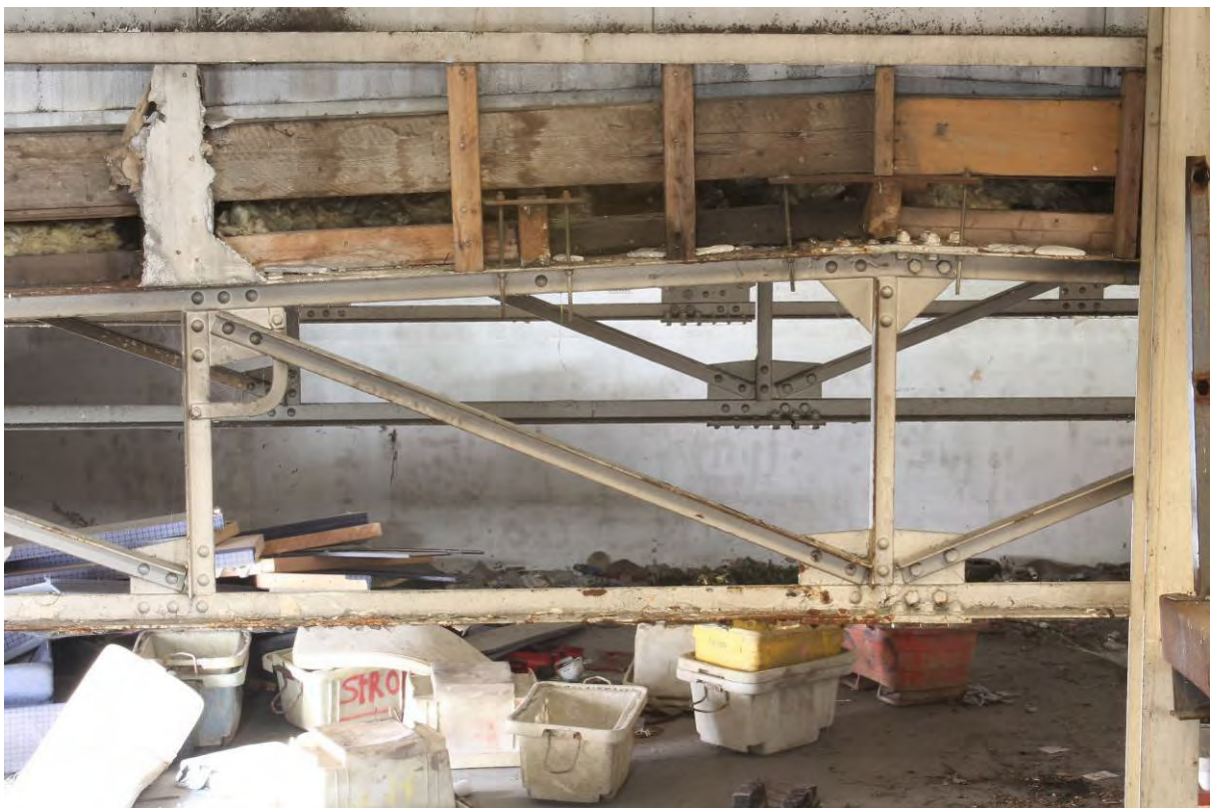
Plate 36 Detail of roof structure above GF7 in Tidal Basin Road Post and Sorting Office, looking south
