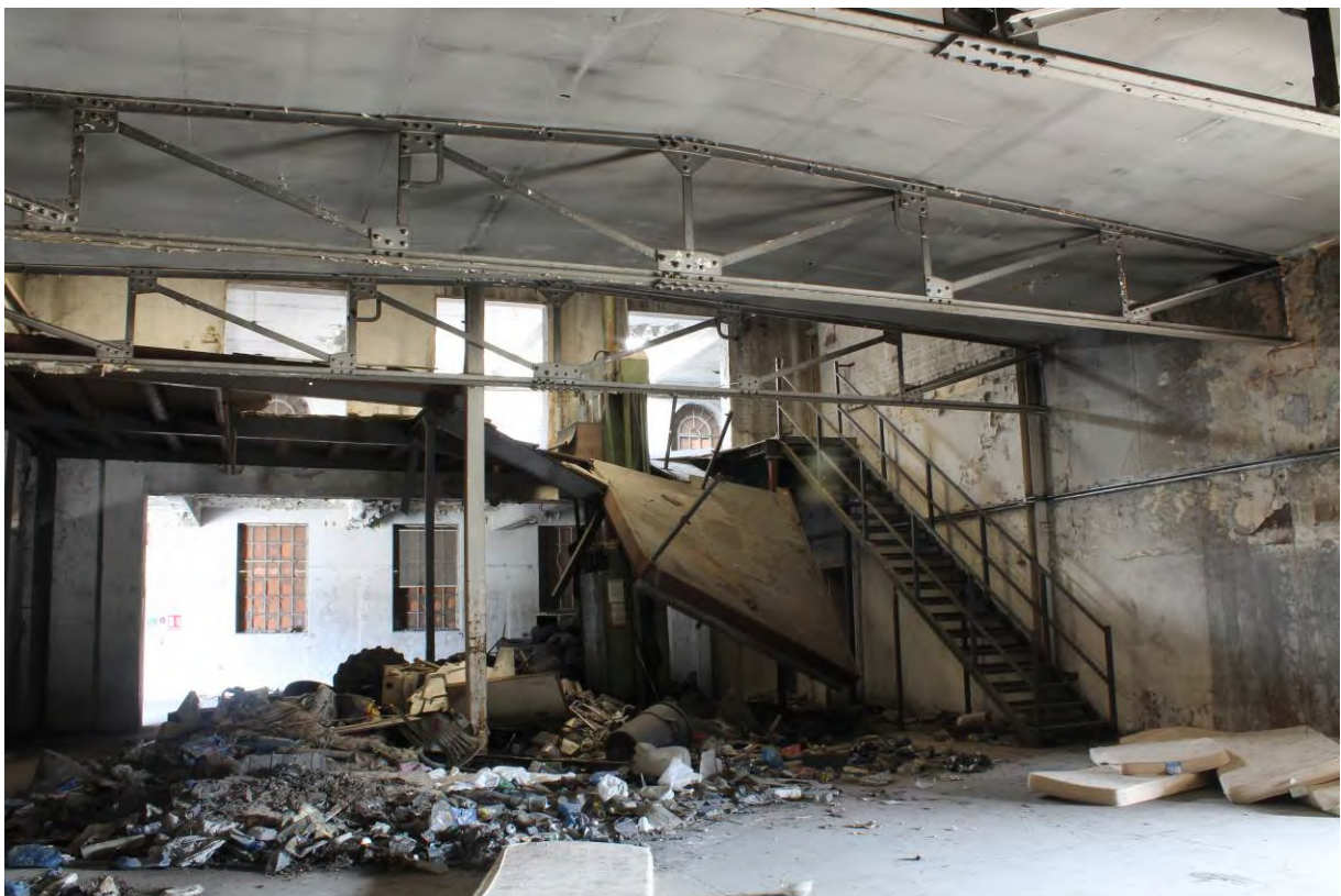
Plate 22 Collapsed mezzanine in Tidal Basin Road Post and Sorting Office, looking north from GF7
