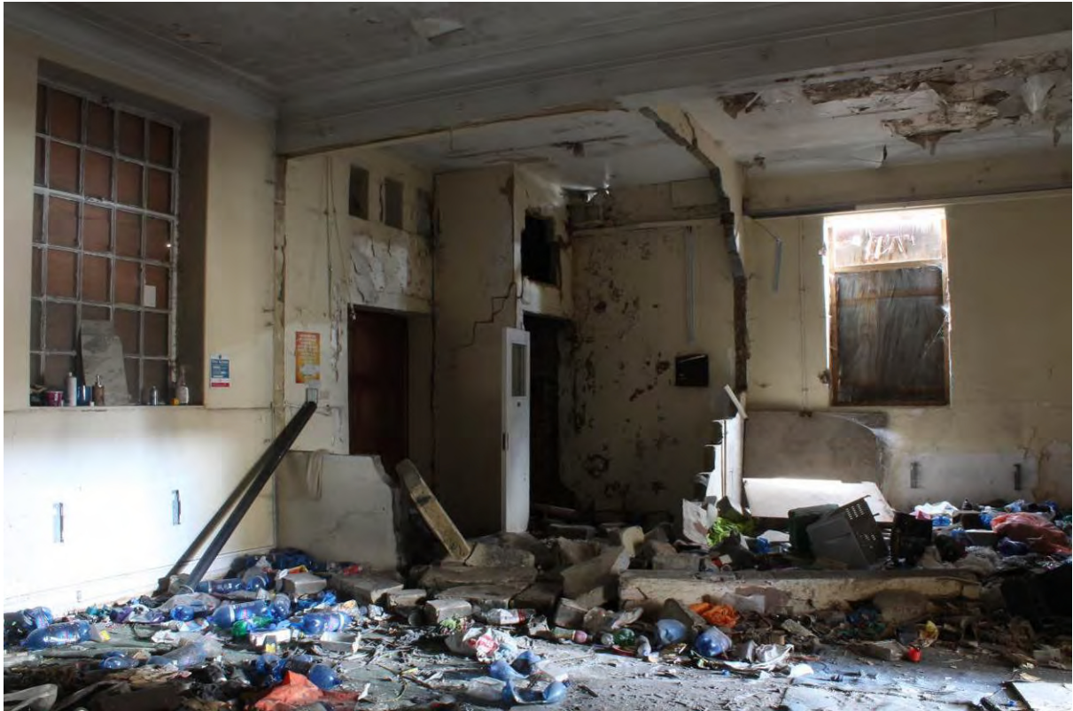
Plate 27 GF2 (former Public Office) in Tidal Basin Road Post and Sorting Office, looking north-east
