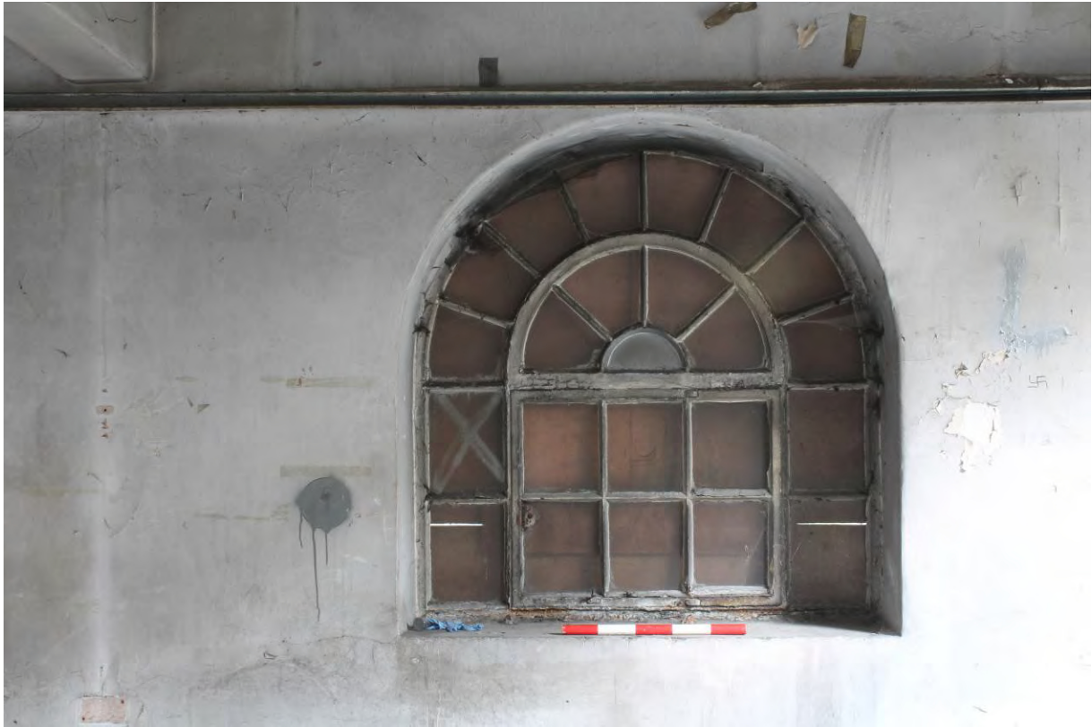
Plate 32 First floor window in the north wall of FF1 in Tidal Basin Road Post and Sorting Office, looking north
