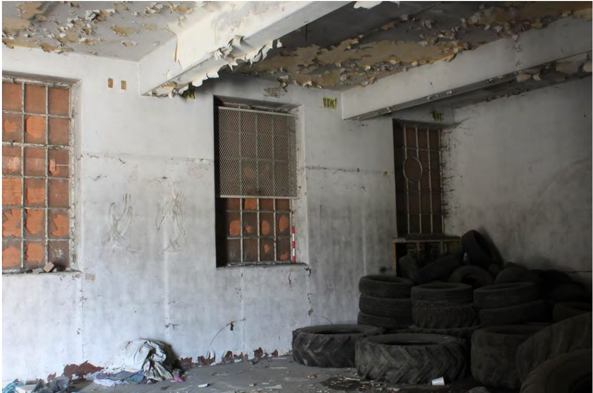
Plate 21 Western bays of GF1 in Tidal Basin Road Post and Sorting Office, looking north
