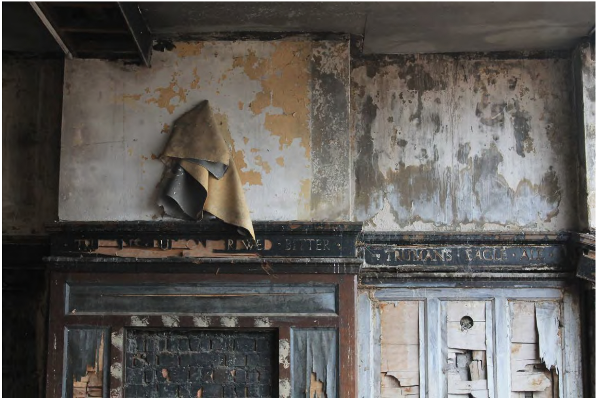
Plate 49 Detail of frieze in Lounge Bar of the Tidal Basin Tavern, looking east
