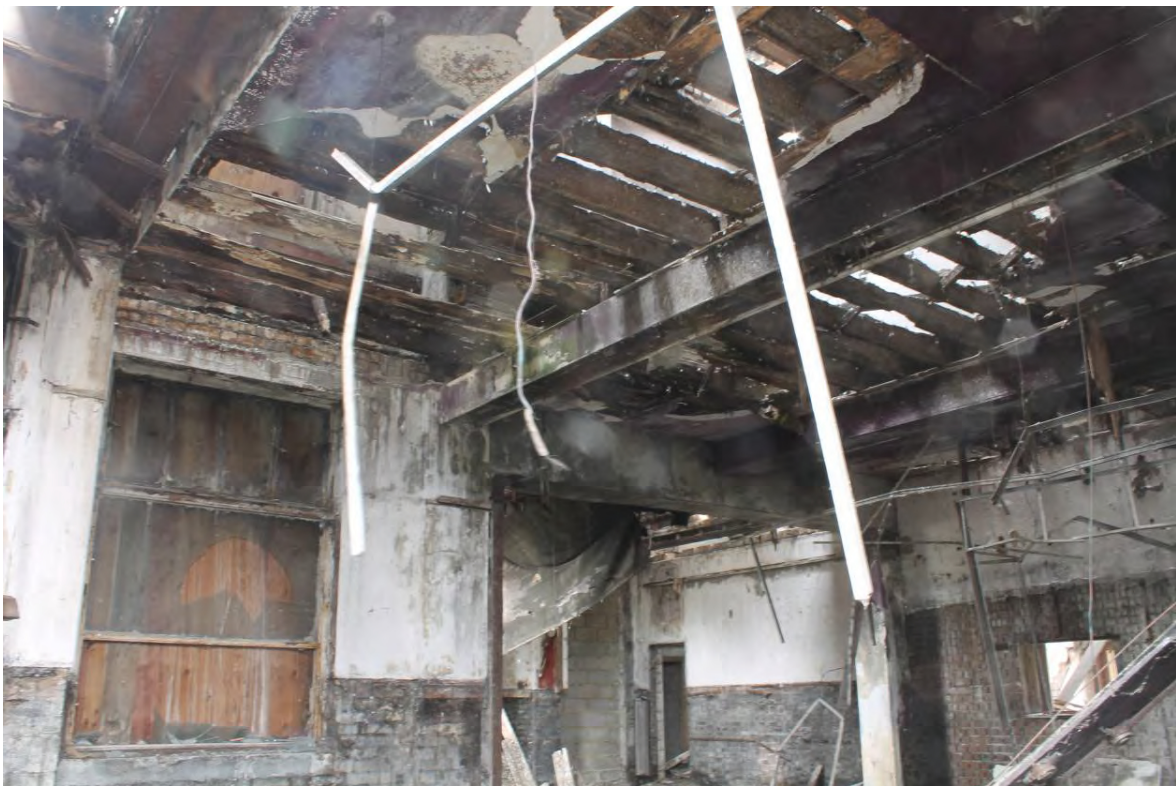
Plate 40 Detail of steel bridging joists over the central part of the front (eastern) bar of Tidal Basin Tavern, looking south-west
