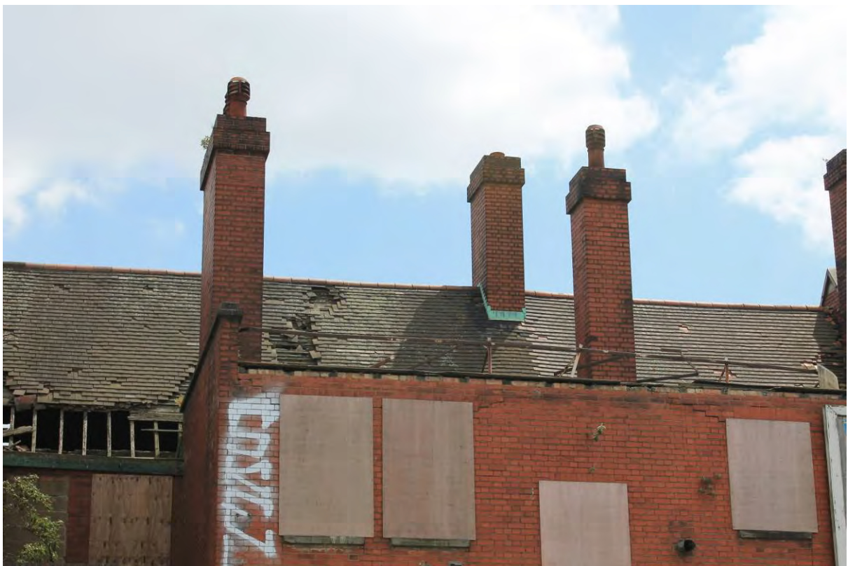
Plate 12 Roofscape and chimney stacks above rear (west) elevation of Tidal Basin Tavern, looking east
