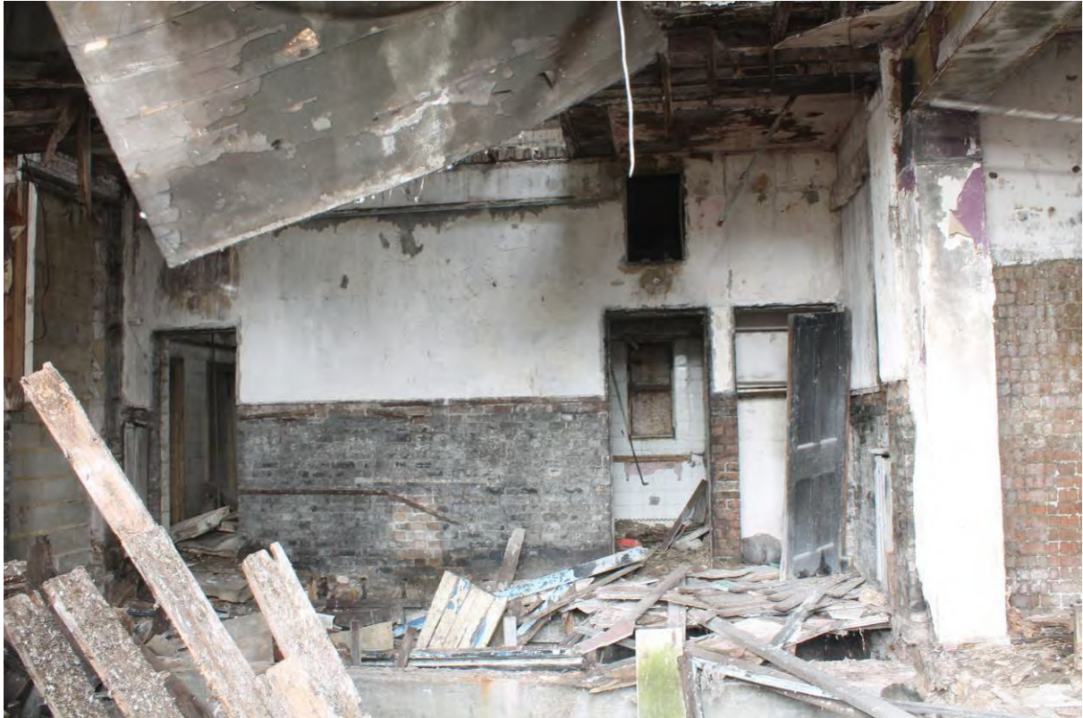
Plate 41 Southern part of the front (eastern) bar of Tidal Basin Tavern, looking west
