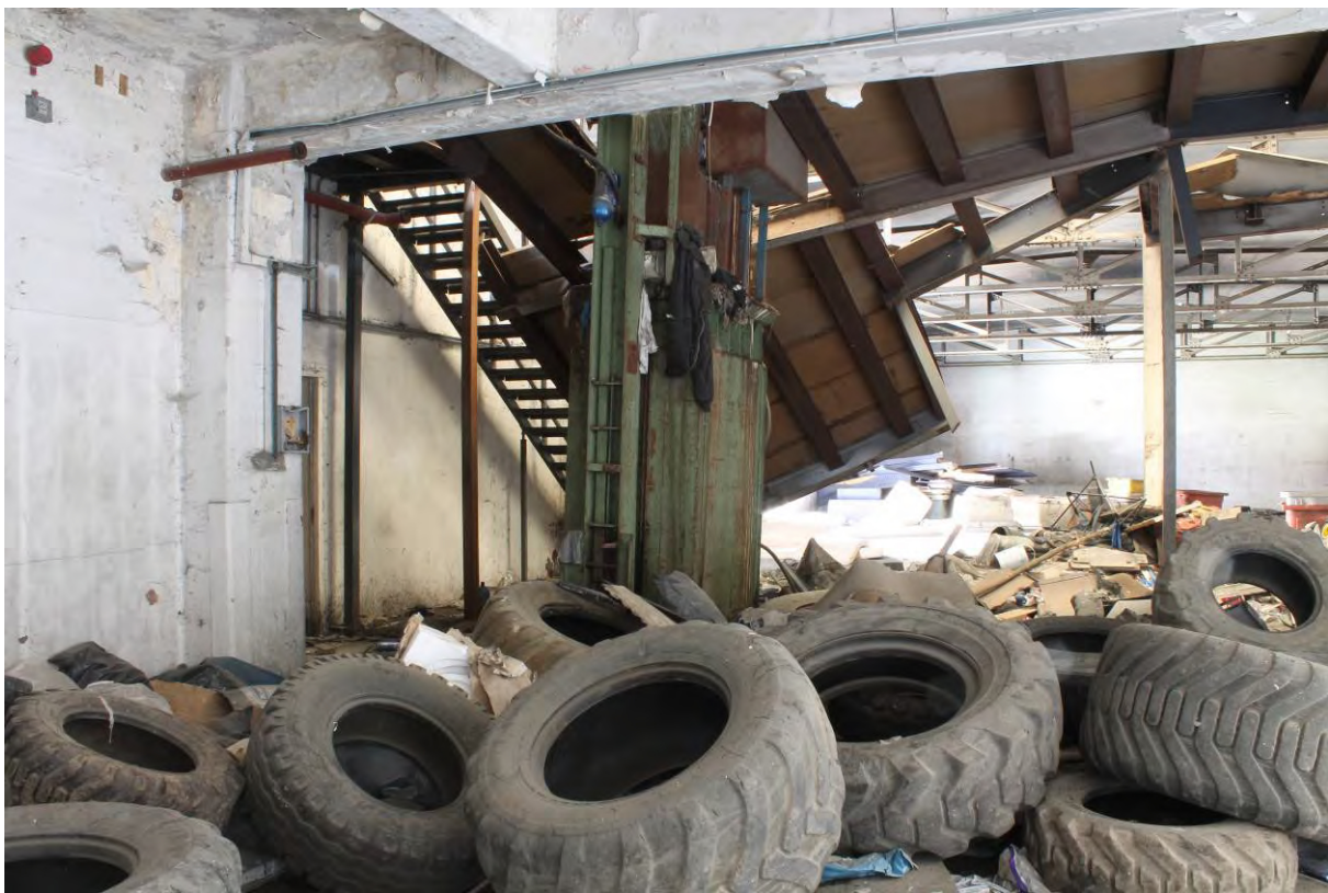
Plate 26 Hydraulic press and collapsed mezzanine in Tidal Basin Road Post and Sorting Office, looking south from GF1 to GF7
