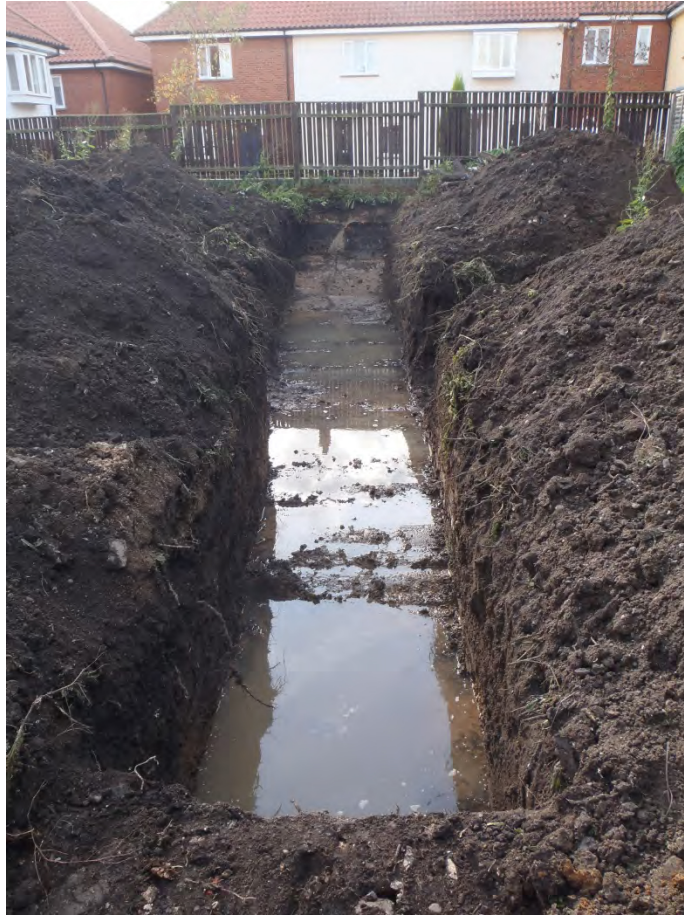
Plate 3: Southeast view of trench showing waterlogged conditions
