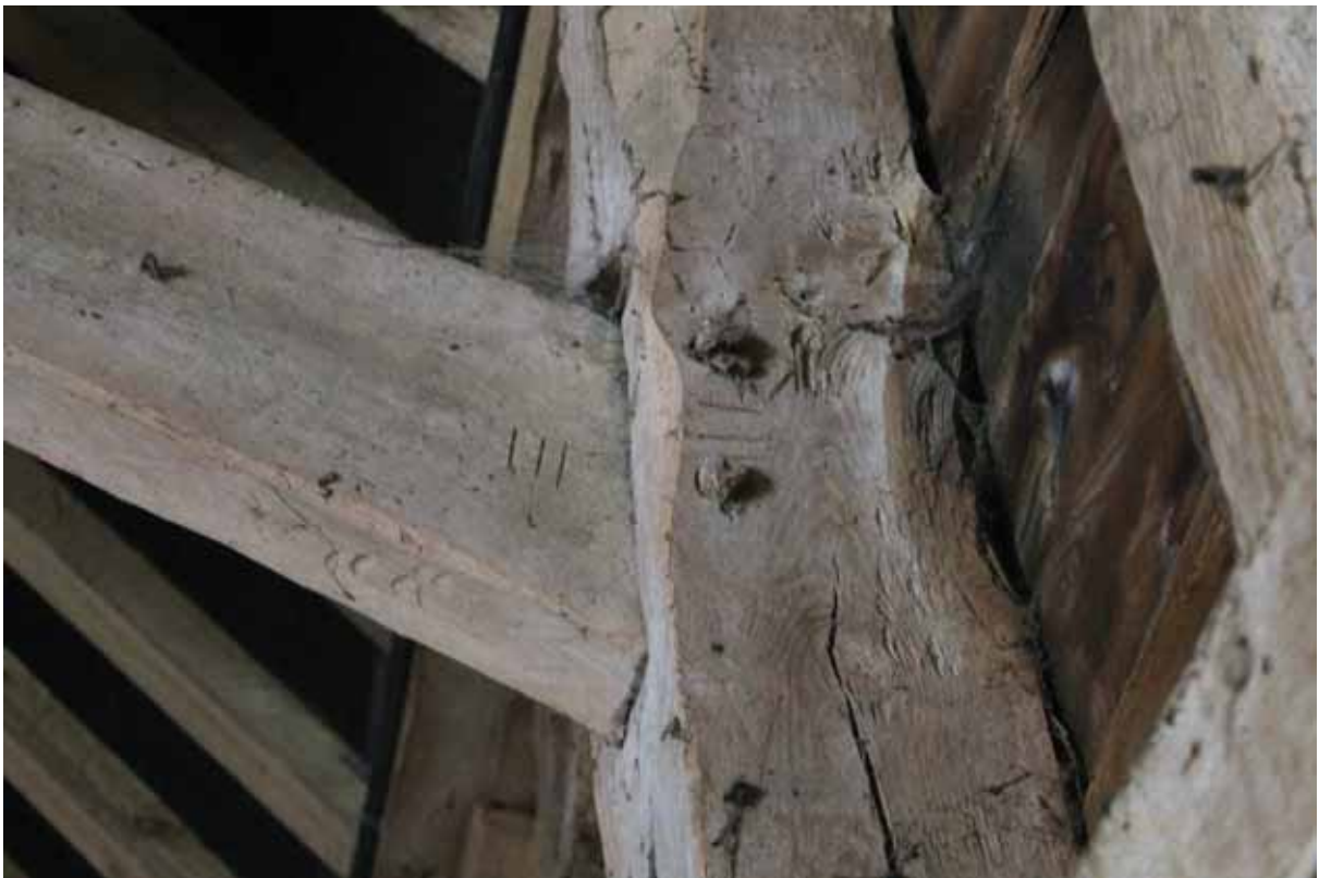
Plate 27 Carpentry marks (III) on wall post and brace of Bay E1/2 in the south-eastern extension, looking south-west
