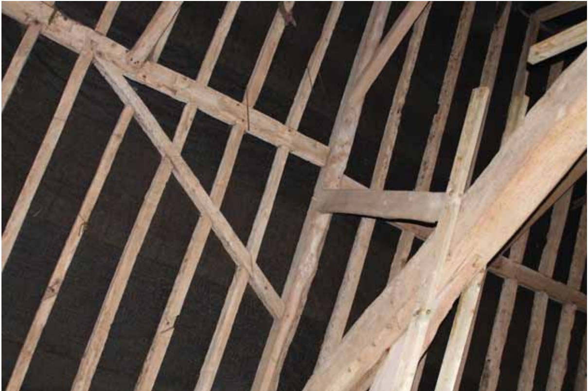
Plate 28 Joggled butt purlin roof in eastern roof pitch of Bays E1/E2 of the south-eastern extension, looking south-east
