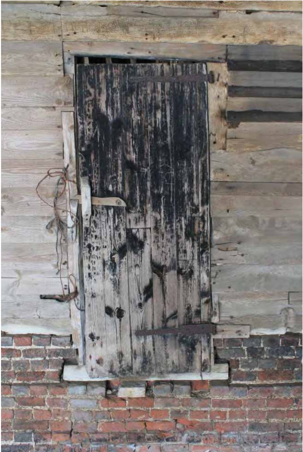
Plate 6 Door in south wall of the main barn under the open fronted shelter, looking north
