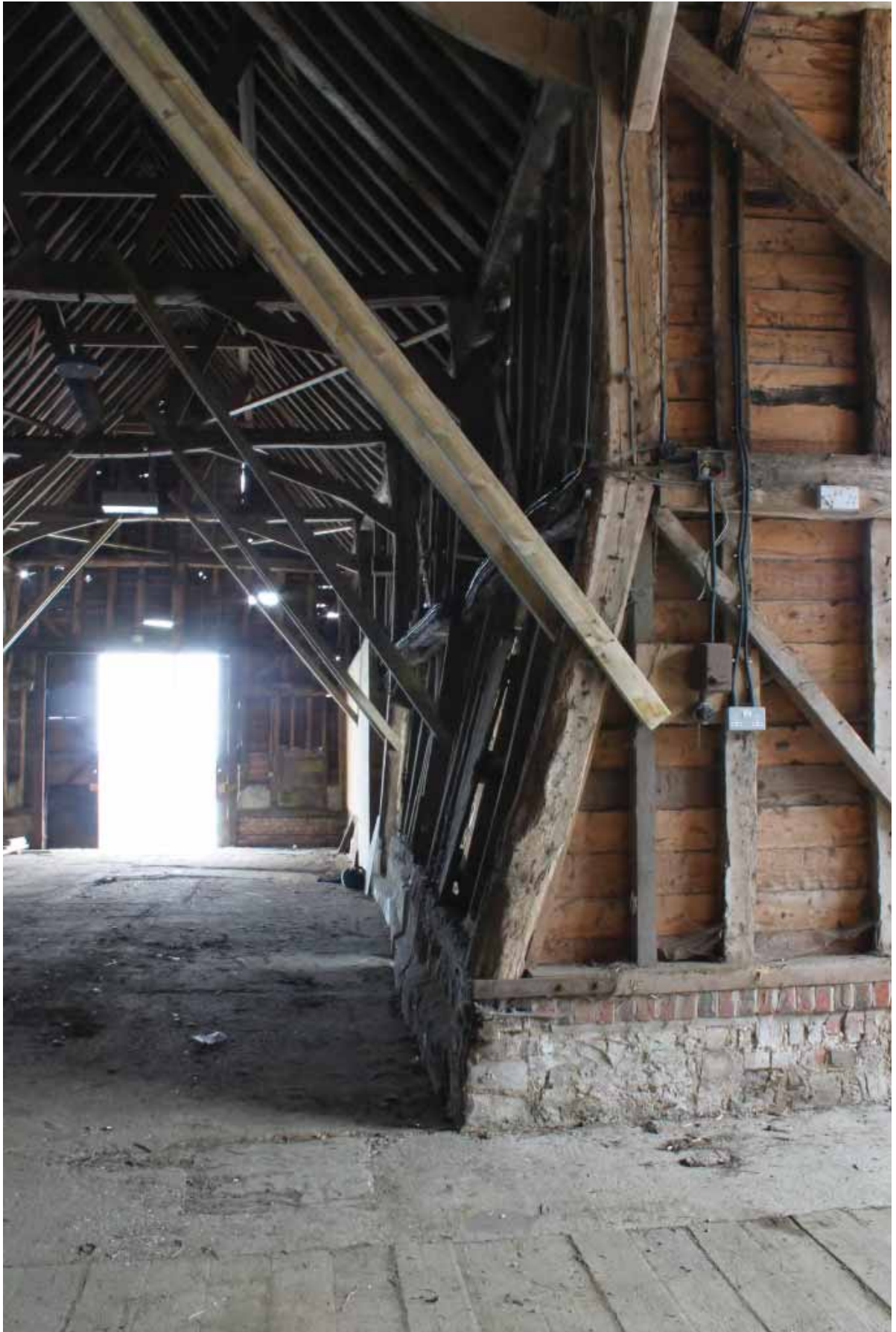
Plate 14 Deformation of wall post (Bay 4/5) and wall frame, looking east
