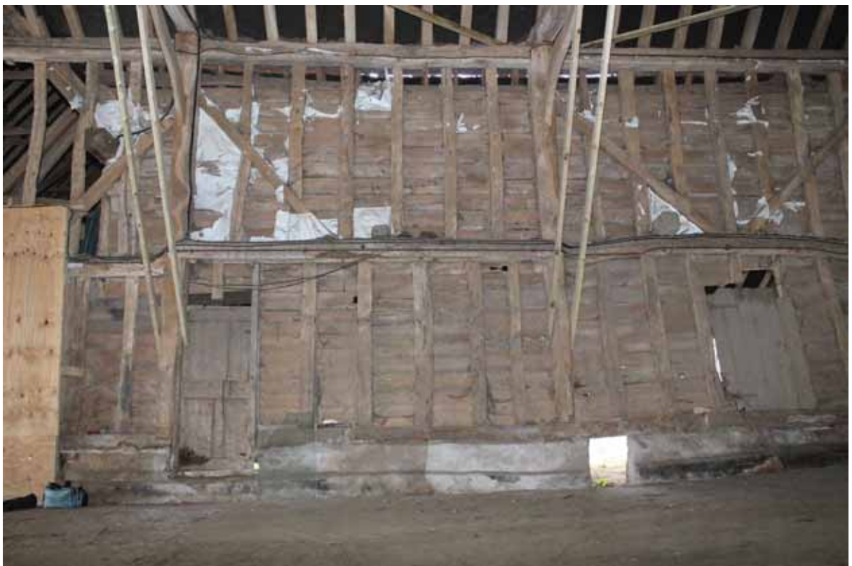
Plate 21 Southern wall frame at Bays 2 (left), 3 (centre) and 4 (right) showing misaligned studding, looking south
