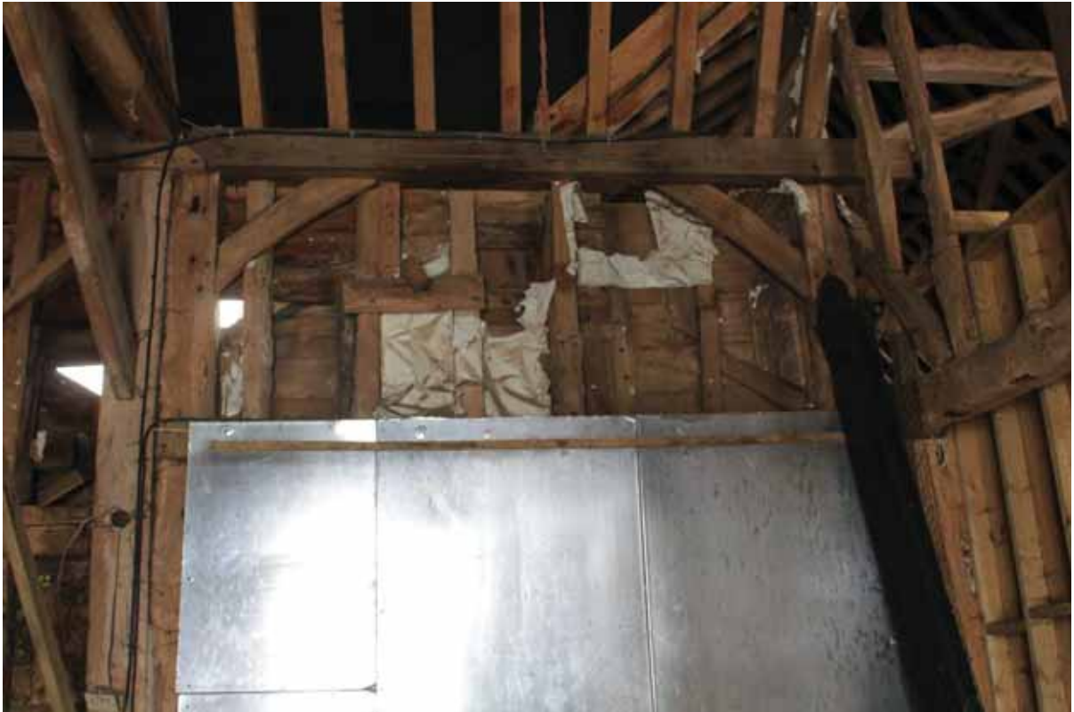
Plate 24 Blocked cart door in western wall of Bay E3 in the south-eastern extension, looking west
