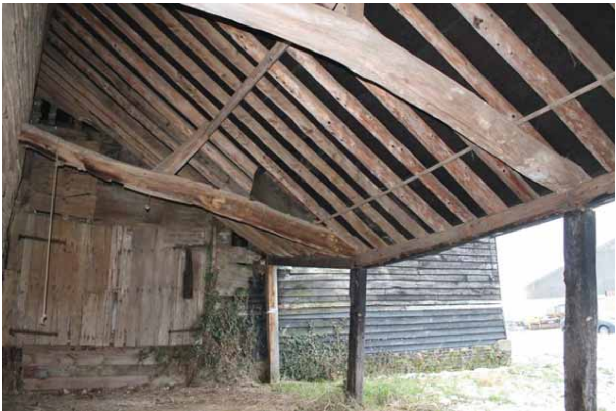
Plate 4 Open fronted shelter showing blocked cart door, looking east
