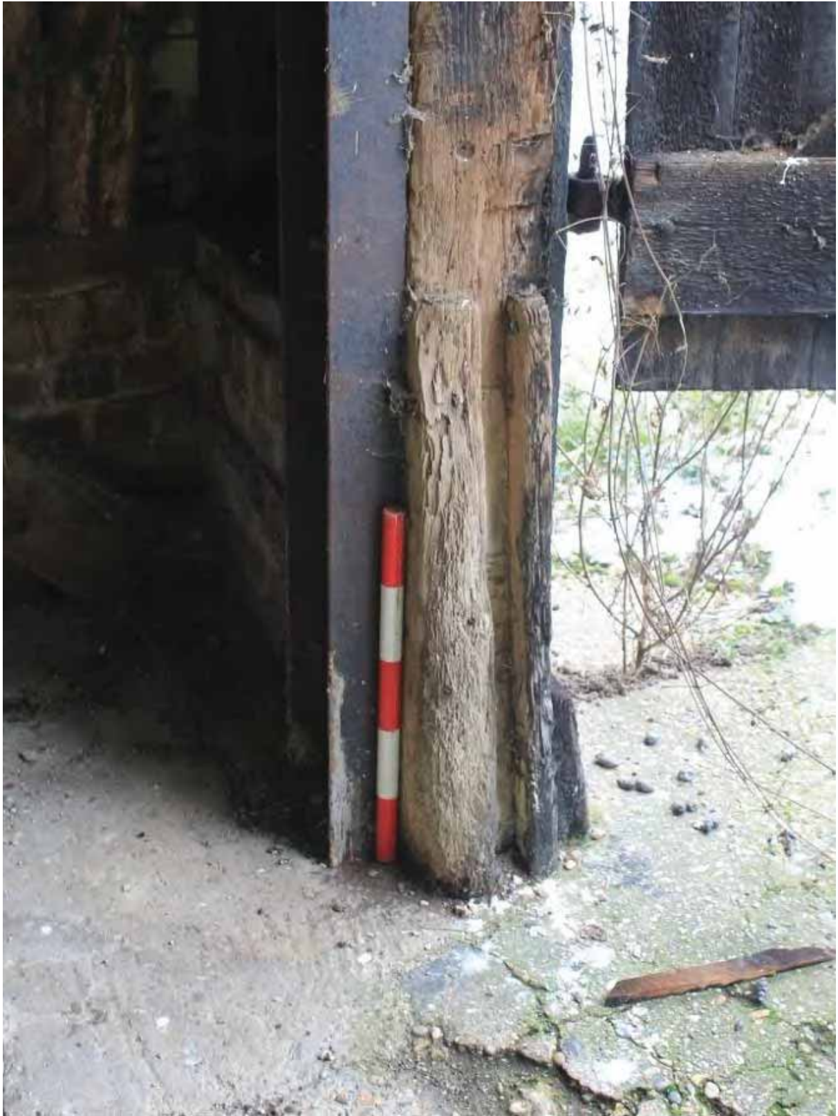
Plate 8 Rebates for leap boards in the east post to the entrance of the midstrey, looking south-east
