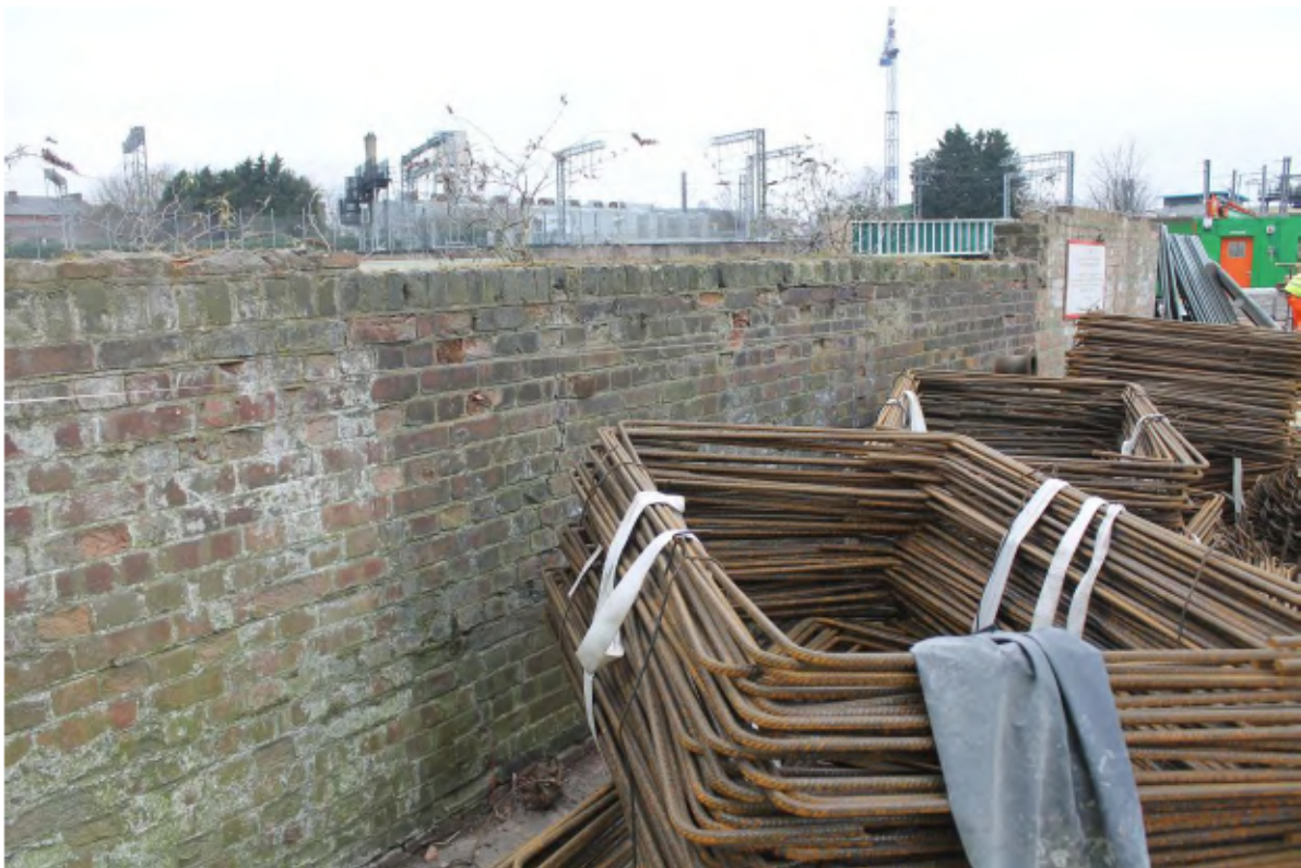
Plate 10: North-east (land) side of the north canal wall showing rebuilt Fletton brick wall, looking north-west towards Point N
