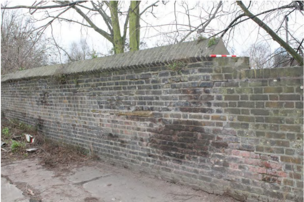
Plate 7: North-east (land) side of the north canal wall at Point M, looking south-east towards Pont L
