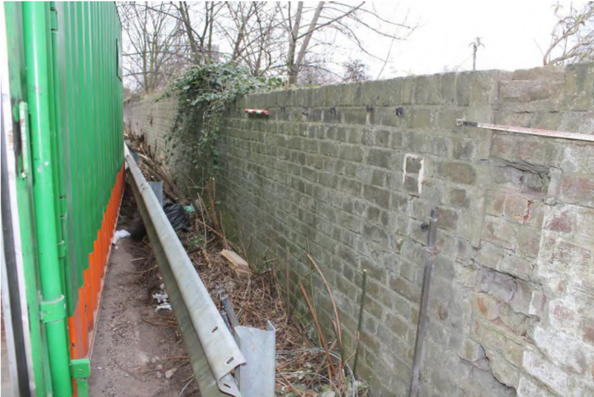
Plate 9: North-east (land) side of the north canal wall showing rebuilt yellow stock brick wall, looking south-east towards Point M
