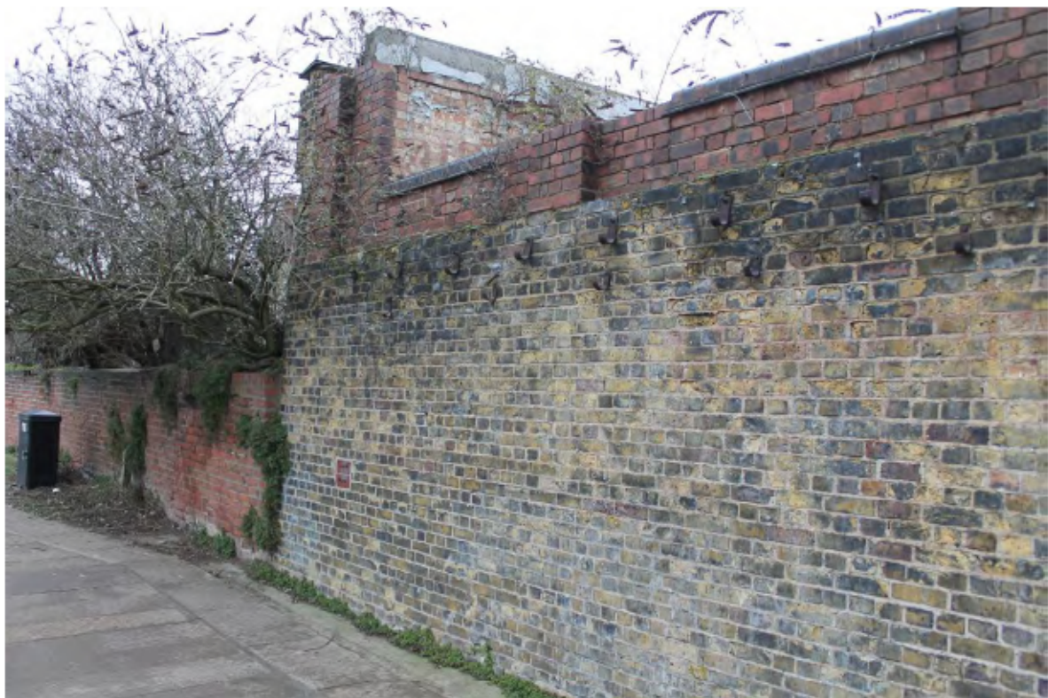
Plate 16: South-west (canal) side of the north canal wall showing overlying Fletton brick wall with integral pilasters and bases of openings looking north-west to Point O and beyond
