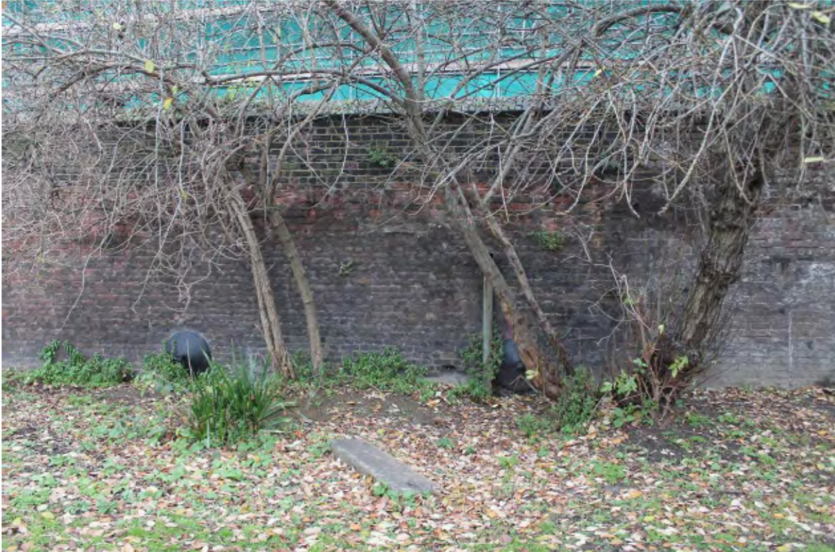
Plate 2: Tie-bar plates at the base of the south-west (canal) side of the north canal wall next to St Pancras Lock (between Points L and M), looking north-east
