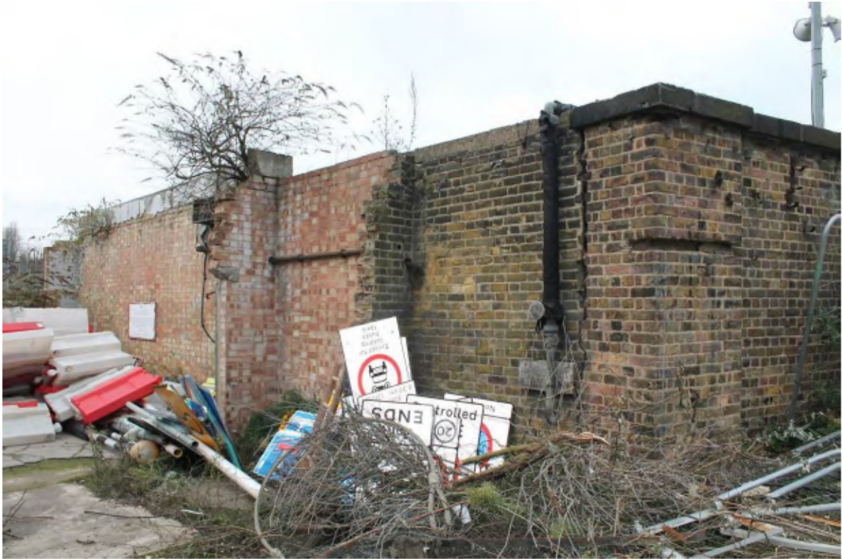
Plate 19: Pier (right) at Point P and remains of Fletton brick building, looking west towards Point O (left)
