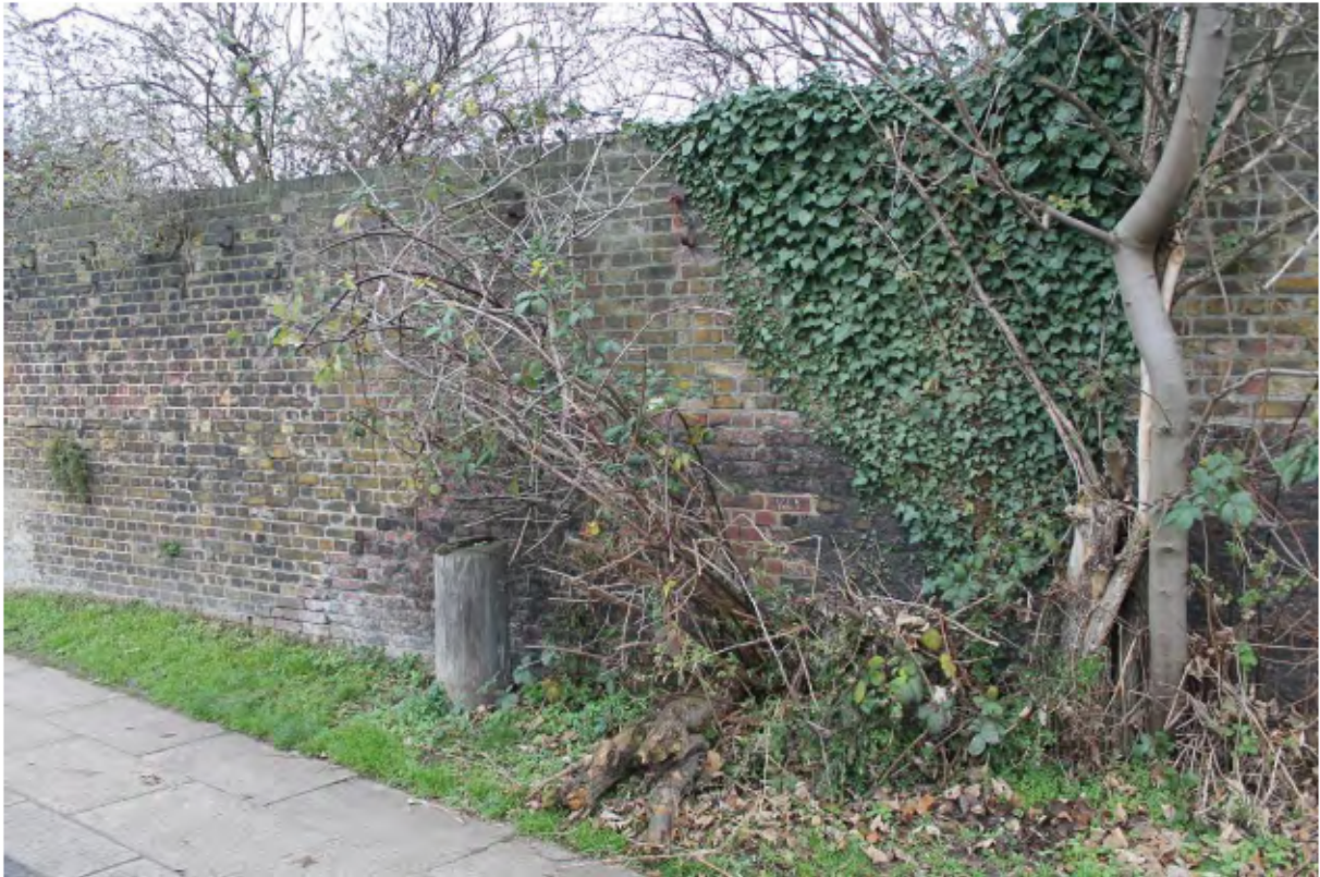
Plate 11: South-west (canal) side of the north canal wall with full height yellow stock brick wall (left), looking north-west towards Point N
