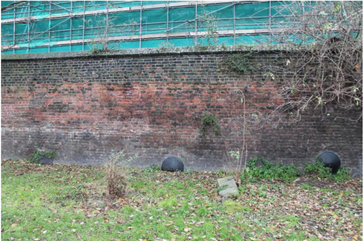
Plate 3: Tie-bar plates and scarring of former building on the south-west (canal) side of the north canal wall next to St Pancras Lock (between Points L and M), looking north-east
