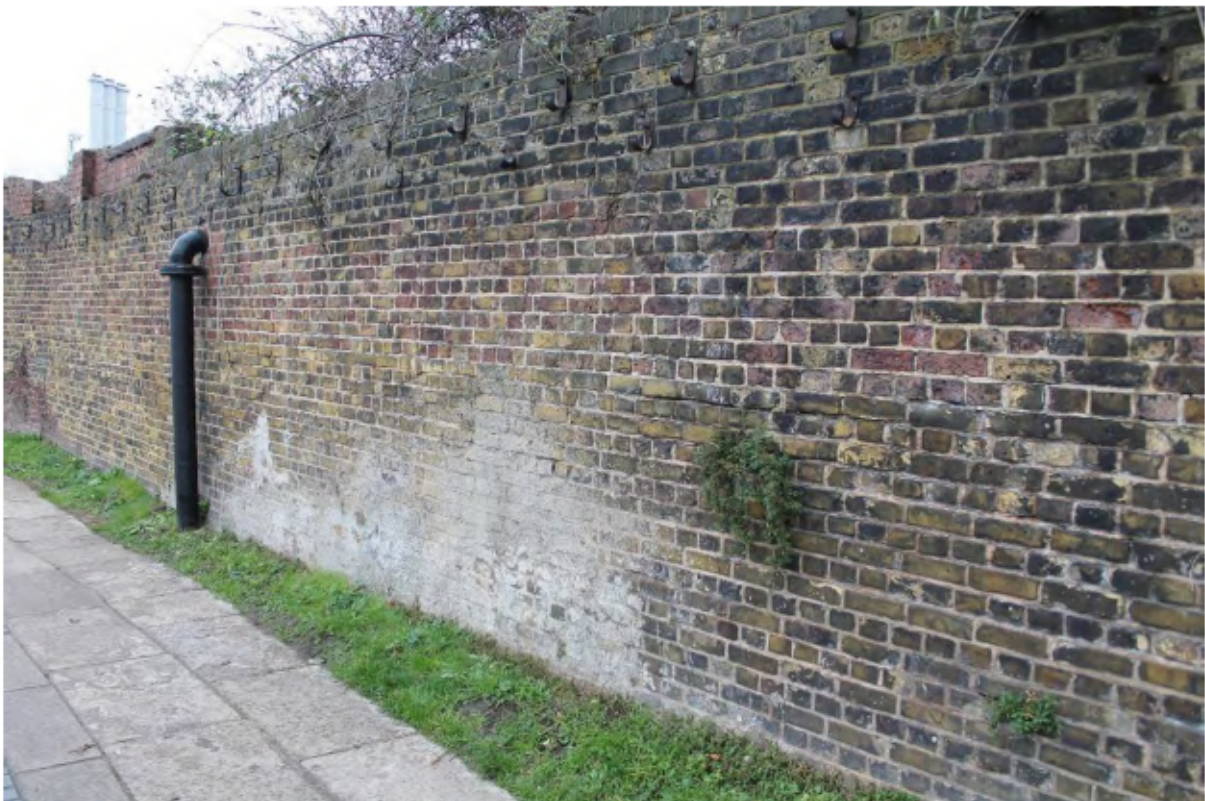
Plate 12: South-west (canal) side of the north canal wall showing 1951 water suction pipe looking north-west towards Point N (near the pipe) and beyond
