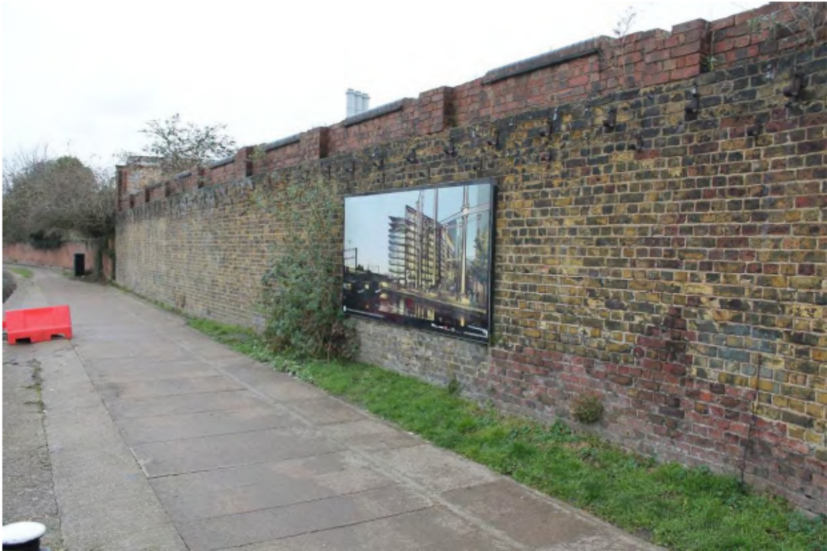
Plate 15: South-west (canal) side of the north canal wall showing overlying Fletton brick wall with integral pilasters and bases of openings looking north-west from Point N towards Point O and beyond
