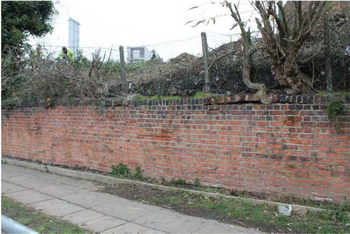
Plate 21: South-west (canal) side of the low red brick north canal wall with chain-link fence above, looking north between Point O and the CTRL Bridge
