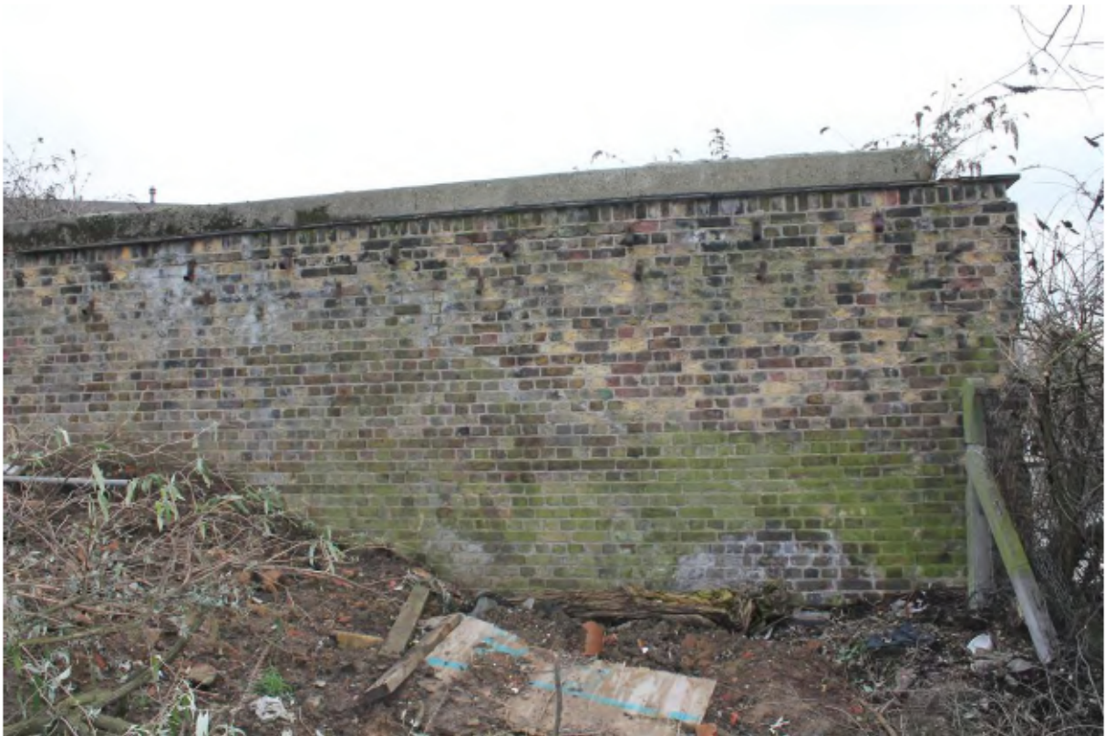
Plate 17: North-west side of return wall (Point O (right) to Point P (to the left), looking south-east
