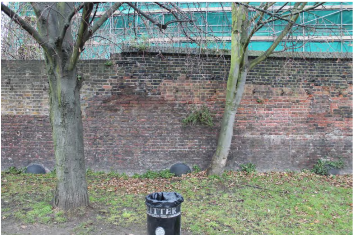
Plate 6: South-west (canal) side of the north canal wall with later rebuilding of the upper part of the wall (left), looking north-east at Point M
