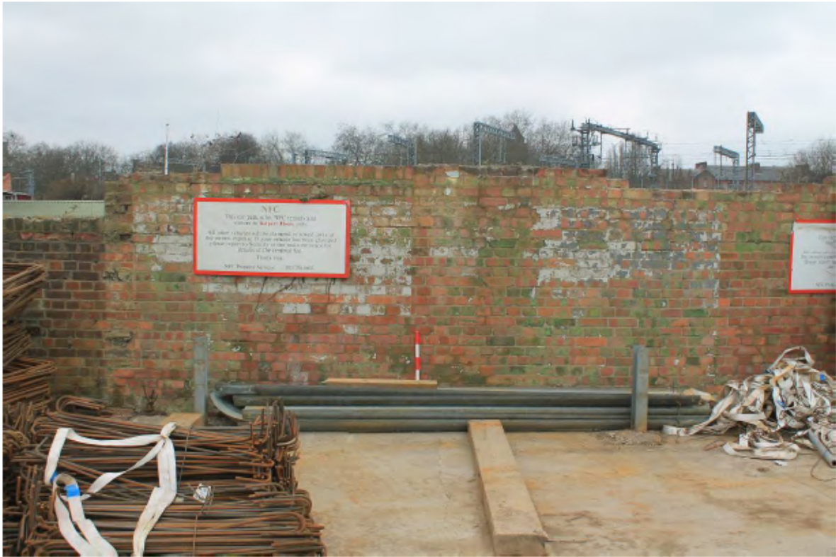
Plate 13: North-east (land) side of the north canal wall showing rebuilt Fletton brick wall, looking south-west with Point N to the left (south-east)
