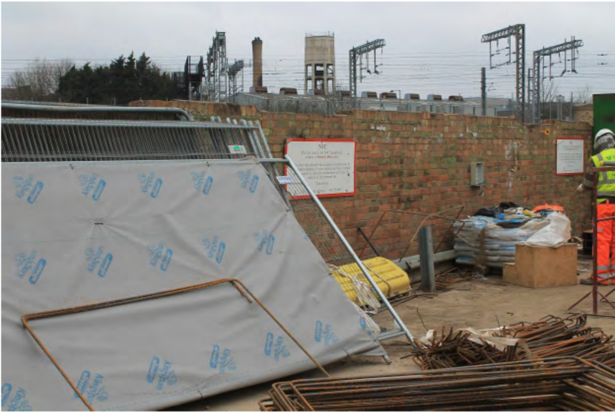
Plate 14: North-east (land) side of the north canal wall showing rebuilt Fletton brick wall, looking west with Point N to the left (south-east) and Point O to the right (north-west)
