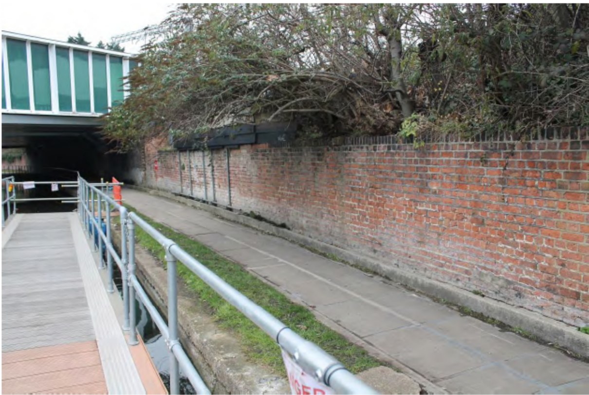
Plate 22: South-west (canal) side of the low brick north canal wall (centre and right) and CTRL Bridge (left) looking north towards Point R
