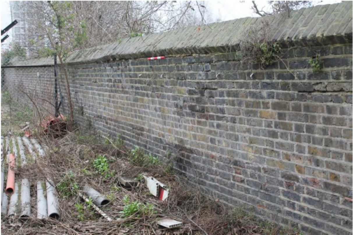
Plate 5: North-east (land) side of the north mid-19th century canal wall, looking south-east from Point M towards Point L
