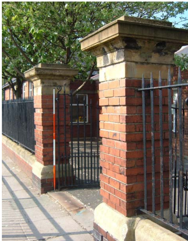
Plate 38. Detail of school gates (northern set) off Sutton Street, from the south-west (2m scale).
