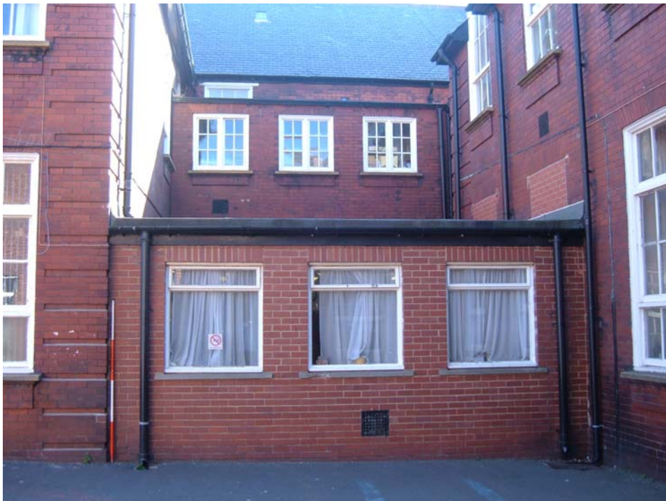
Plate 10. Main building, central range (north), west elevation and hall block, north elevation (east end), from the north-west (2m scale).
