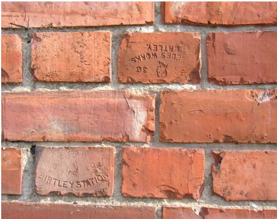
Plate 18. Gym block, north elevation (west end), detail of brick stamps, from the north.
