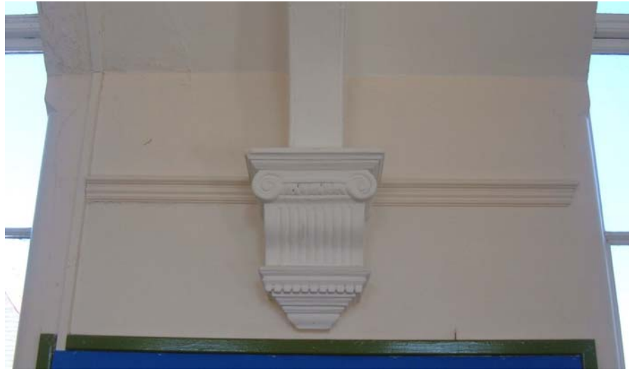
Plate 53. Main building, first floor, detail of impost in upper hall, from the south-east.
