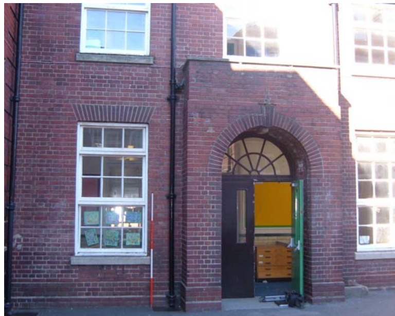
Plate 26. Former secondary modern block, central range, north entrance in west elevation, from the north-east (2m scale).
