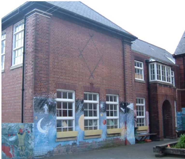
Plate 24. Former secondary modern block, south wing, east elevation, from the south-east (2m scale).
