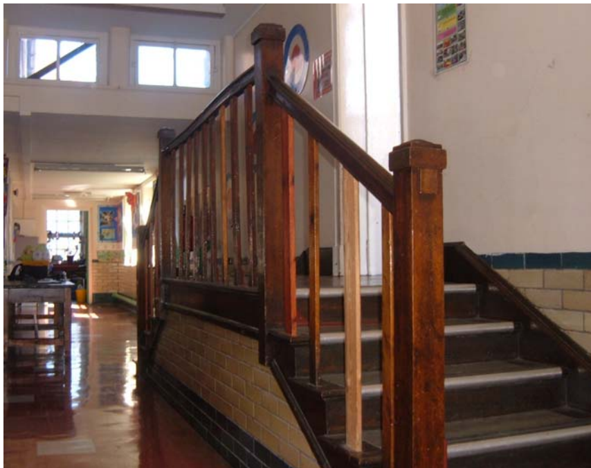
Plate 56. Former secondary modern block, first floor, detail of mezzanine staircase in corridor, from the south.
