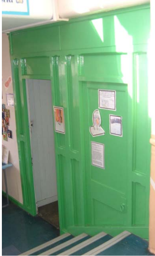
Plate 49. Main building, first floor (north-end), detail of alteration to former cloakroom, from the south-west.
