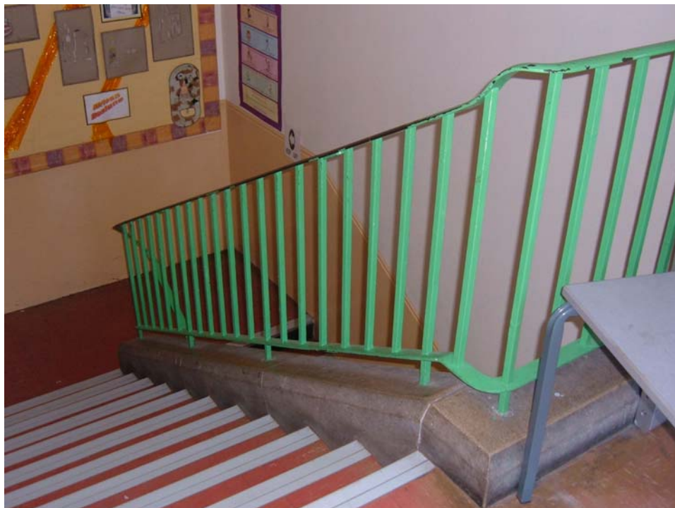
Plate 60. Former secondary modern block, first floor, dog-leg stairs (northern set), from the east.
