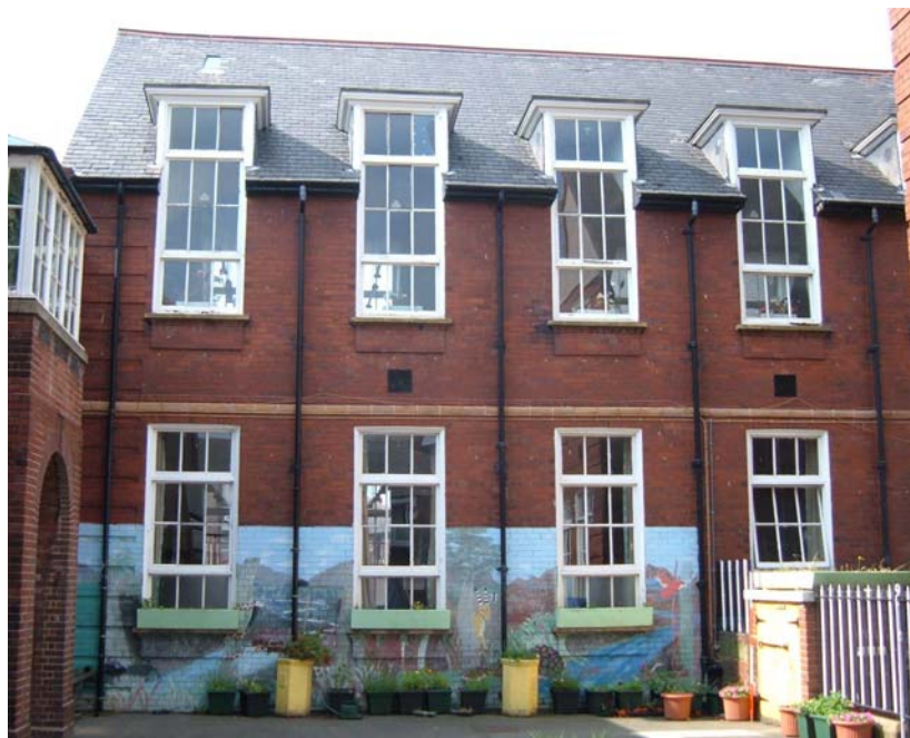
Plate 8. Main building, hall block, south elevation (west end), from the south-east (2m scale).
