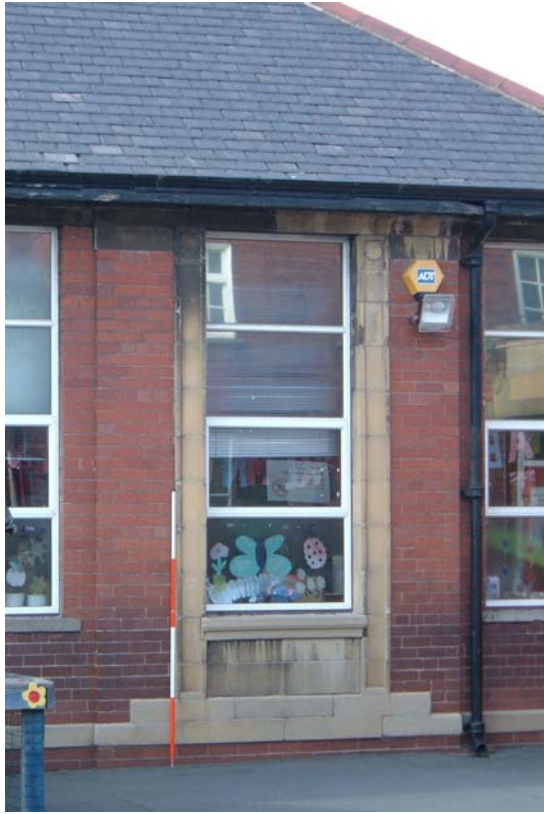
Plate 31. Former infants' block, south elevation (east end), window detail, from the south-east (2m scale).
