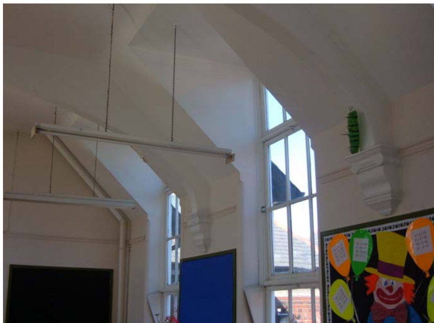
Plate 52. Main building, first floor, detail of roof in upper hall, from the south-east.
