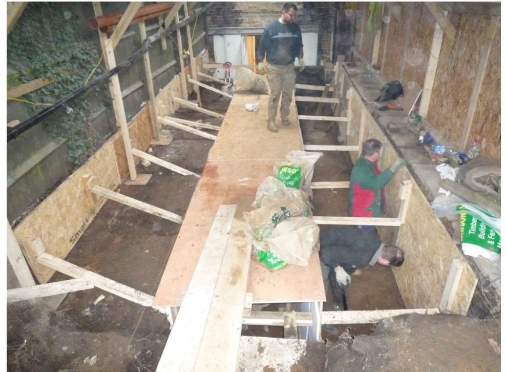
Plate 4: West Facing Shot of Installation of Shoring During Phase 2 Excavation (Natural Gravel Exposed Across Base of Trench)
