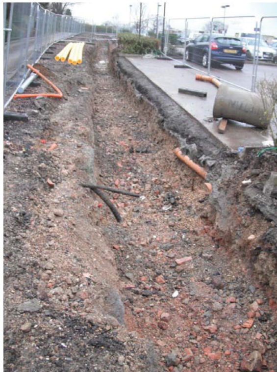
Plate 2: Recent Deposits to Base of trench, Eastern Side of Site, Looking West
