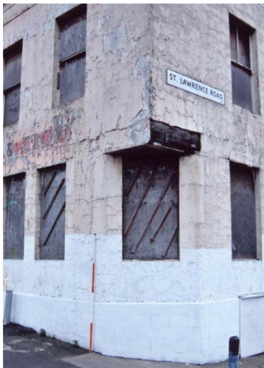
Plate 4. The Rose & Crown, main building, detail at the north-west corner, from the north-west (2m scale)
