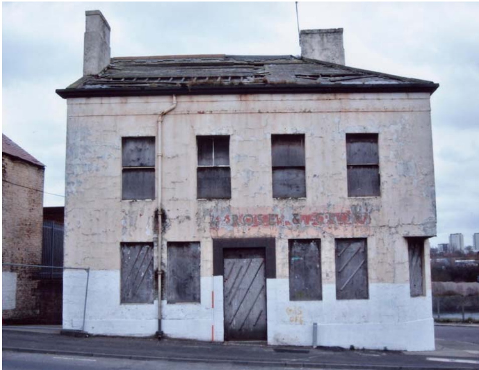
Plate 3. The Rose & Crown, main building, north elevation, from the north (2m scale).
