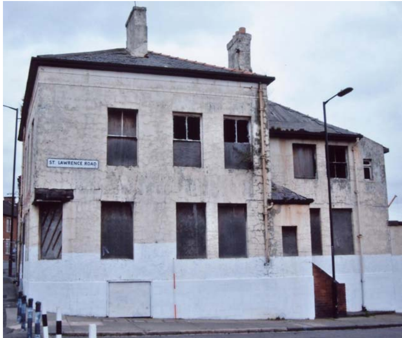
Plate 5. The Rose & Crown, main building, west elevation, from the west (2m scale).
