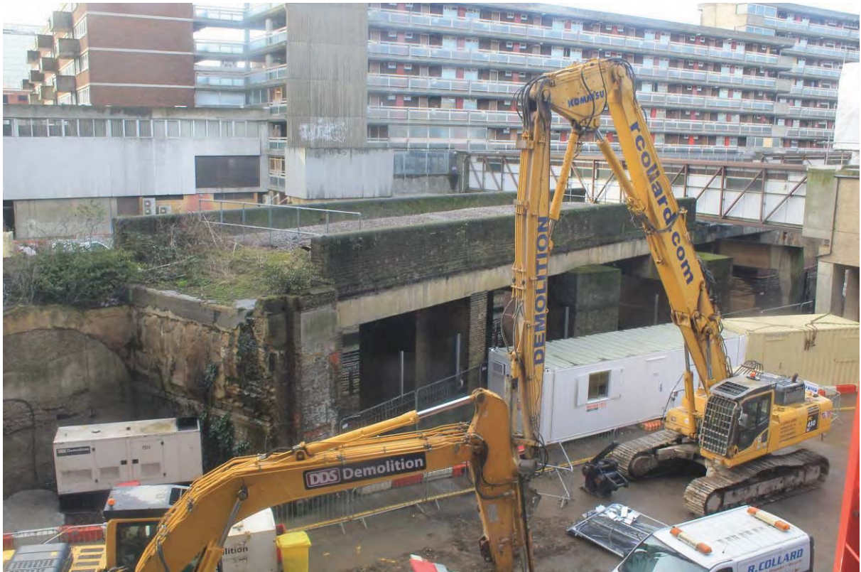
Plate 3: Length of the viaduct rebuilt in the 1920s with concrete beam, looking south-west
