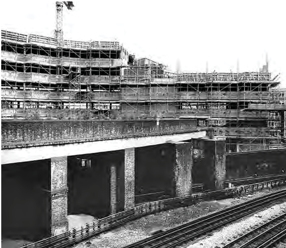
Plate A: Photograph taken in 1980 showing the c.1926 concrete beam bridge section of the viaduct, the northernmost track looping under the viaduct and the construction of West 45 Office Building, looking north-east
