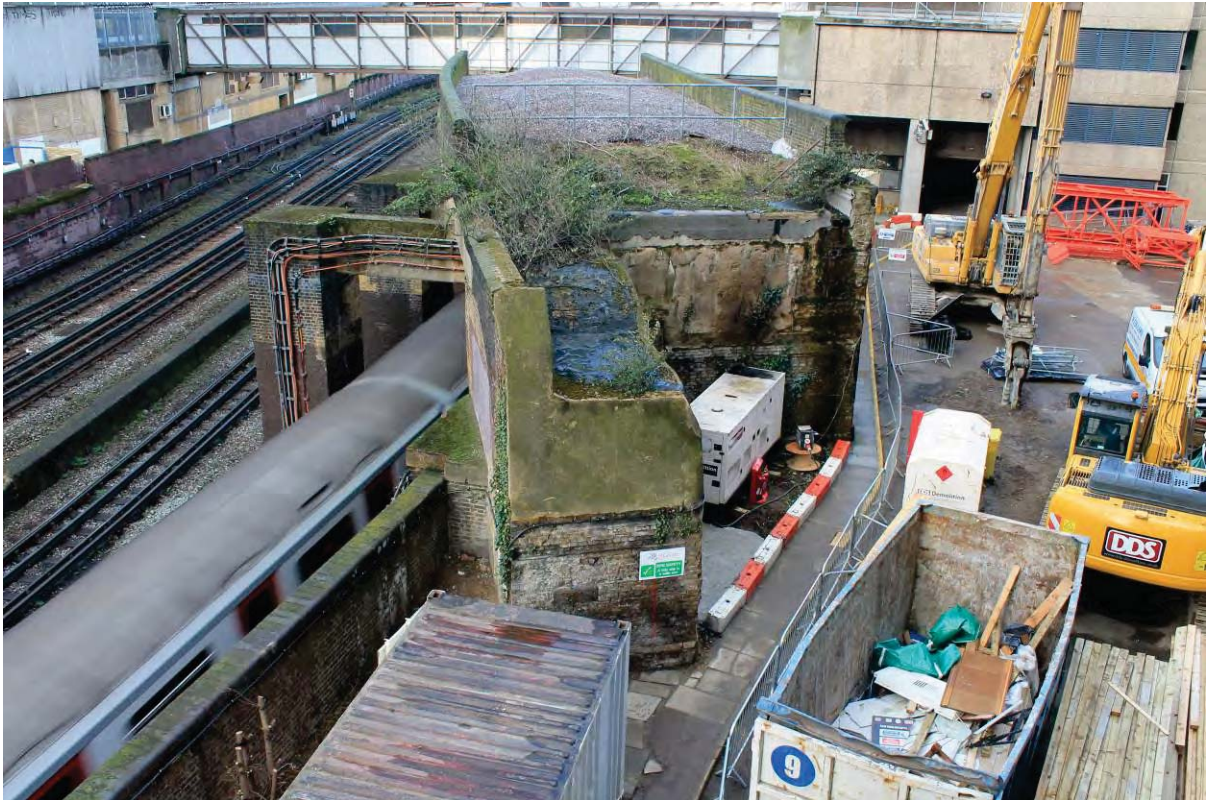
Plate 1: Viaduct and Piccadilly and District railway line, looking west from the 3 rd floor of the West 45 Building
