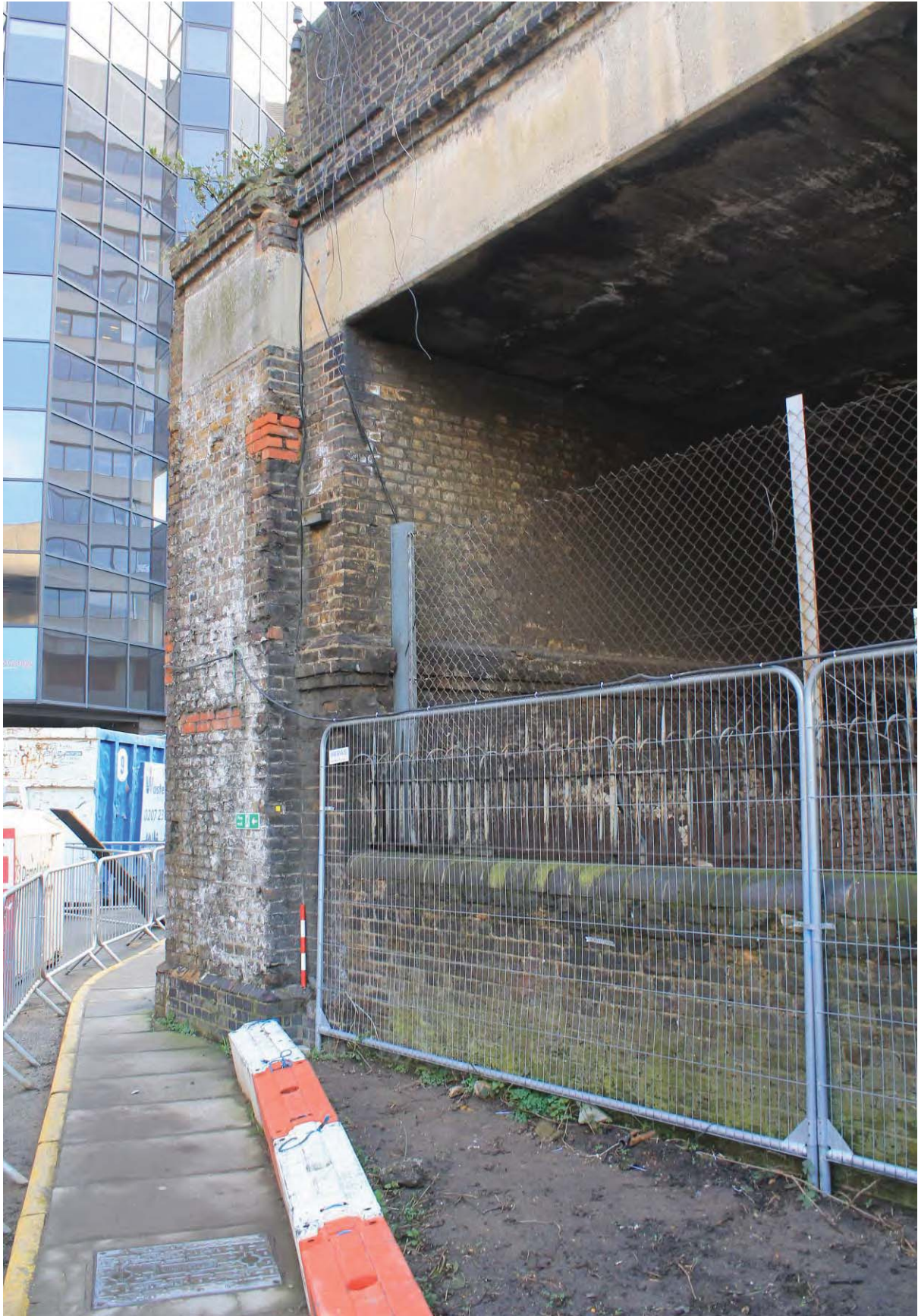
Plate 12: Northern elevation of the 1920s length of viaduct with a rebuilt pier at the junction of the 1869 and 1920s builds, looking south-east
