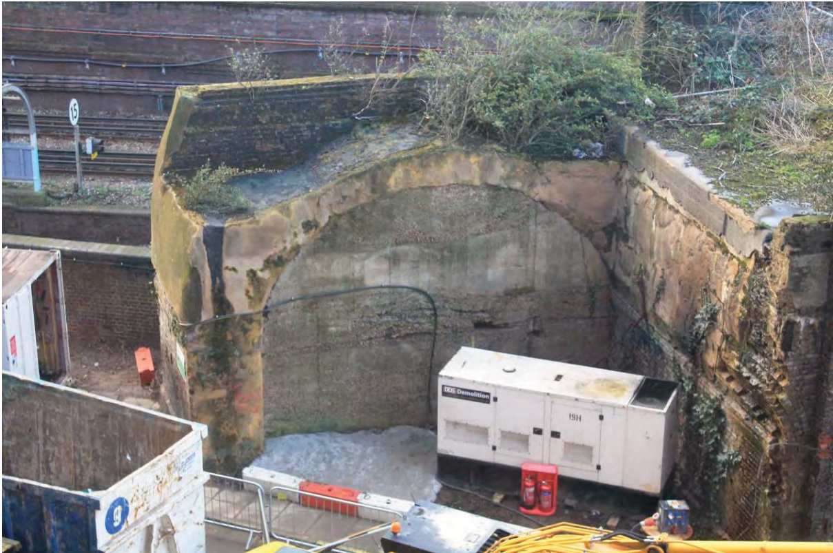
Plate 8: Rendered northern cut back elevation of the eastern end of the remaining viaduct, looking south from West 45 Building
