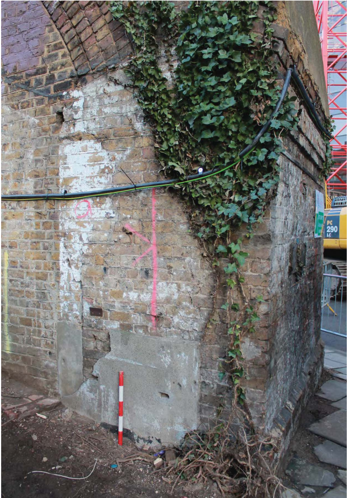
Plate 6: Extent of proposed truncation (to pink line) of the viaduct from eastern end, looking north-west
