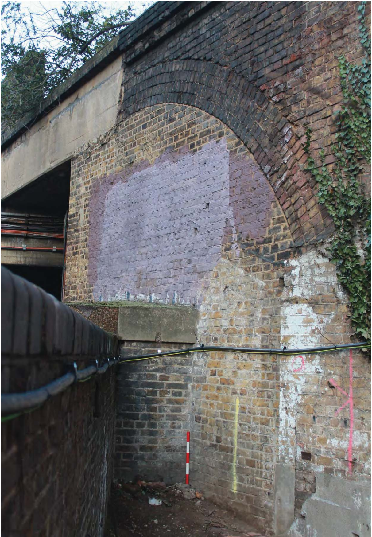
Plate 5: Southern elevation of the viaduct within the site showing later brick blocking, looking west
