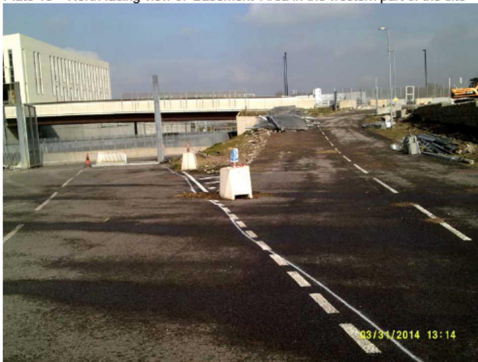
Plate 10 – North facing view of 'Basement' Area in the western part of the site
