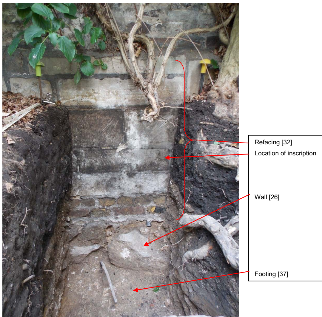
Plate 6: Test Pit 2 viewed south showing wall [26] atop previous footing [37]. The visible brickwork and ashlar coursing above is the 19th century refacing of the wall.
