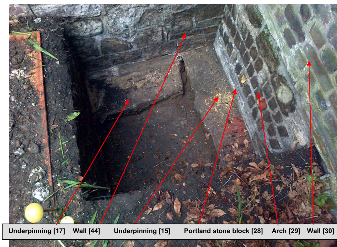
Plate 9: Test Pit 3 viewed east showing 20th century underpinning, prior to deeper excavation
