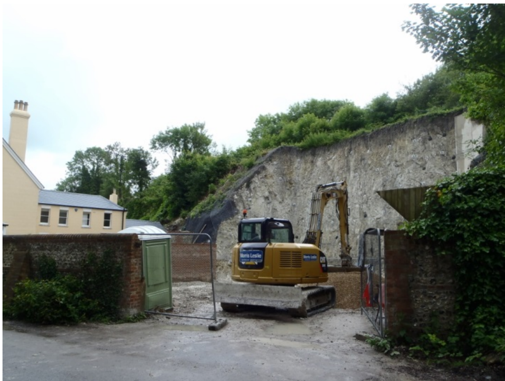
Plate 3: View of site from Domum Road with Wharf House to left. View north-east. Digital image 13.
