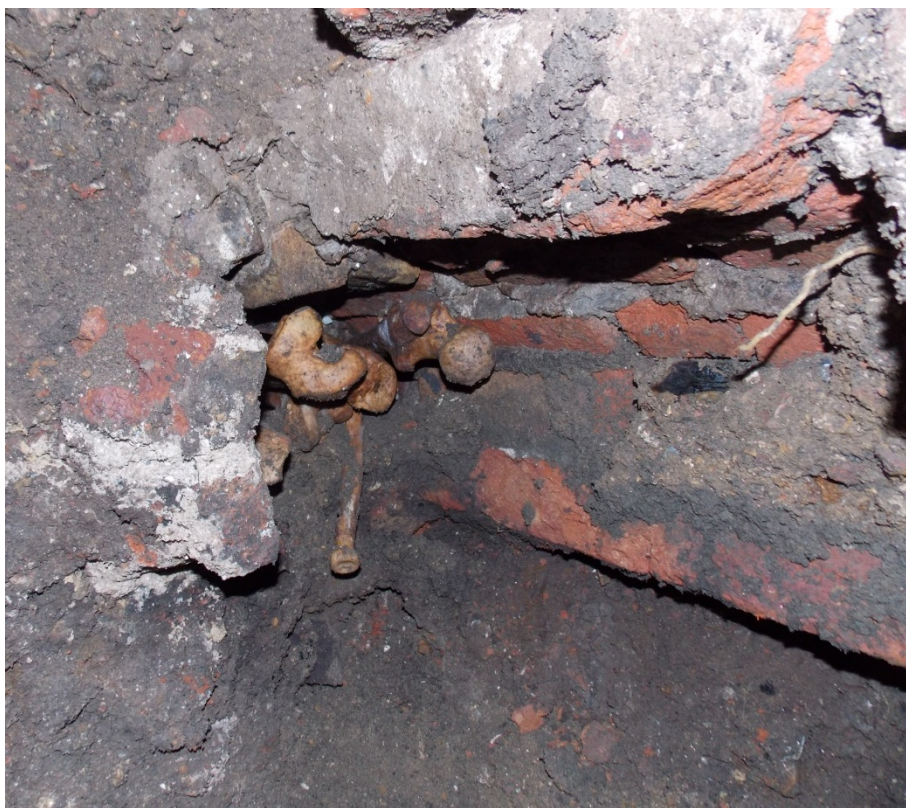
SSW Facing Shot of TP5 Showing Disarticulated Human Remains Within Brick Culvert
