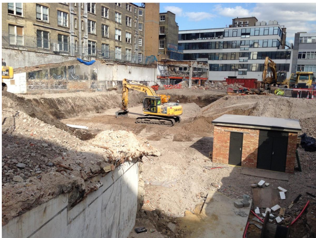
Plate 1: View northeast across northern half of site showing area after reduction to formation level.
