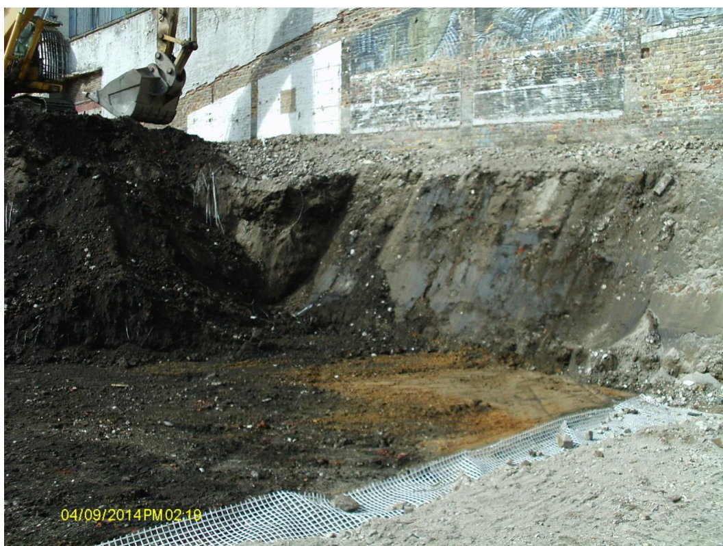
Plate 2: View northeast of ground reduction in progress at northern side of site; the surface of the Hackney Gravels is visible.
