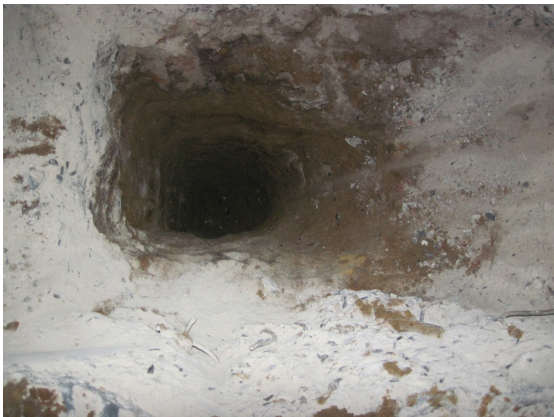
Plate 1 North facing view of Test Pit 1; concrete immediately above natural sands and gravels
