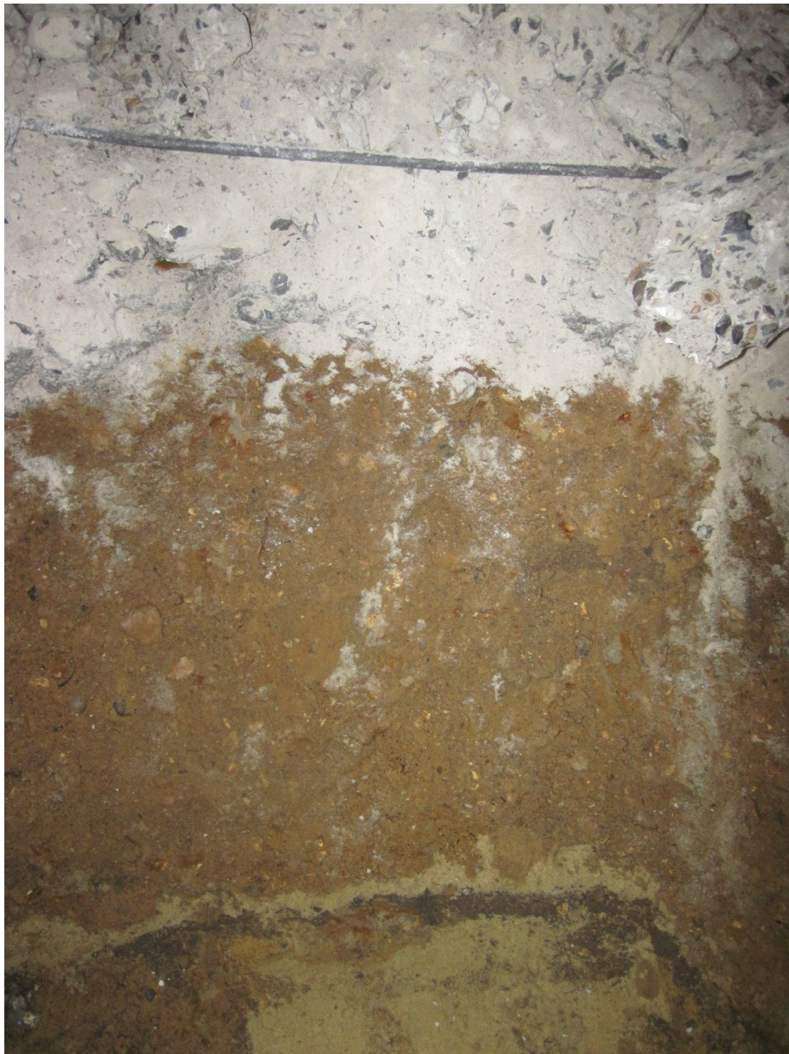
Plate 4 West facing section in Test Pit 4 showing sequence of concrete and re-deposited natural (+) above concrete encountered at excavation depth
