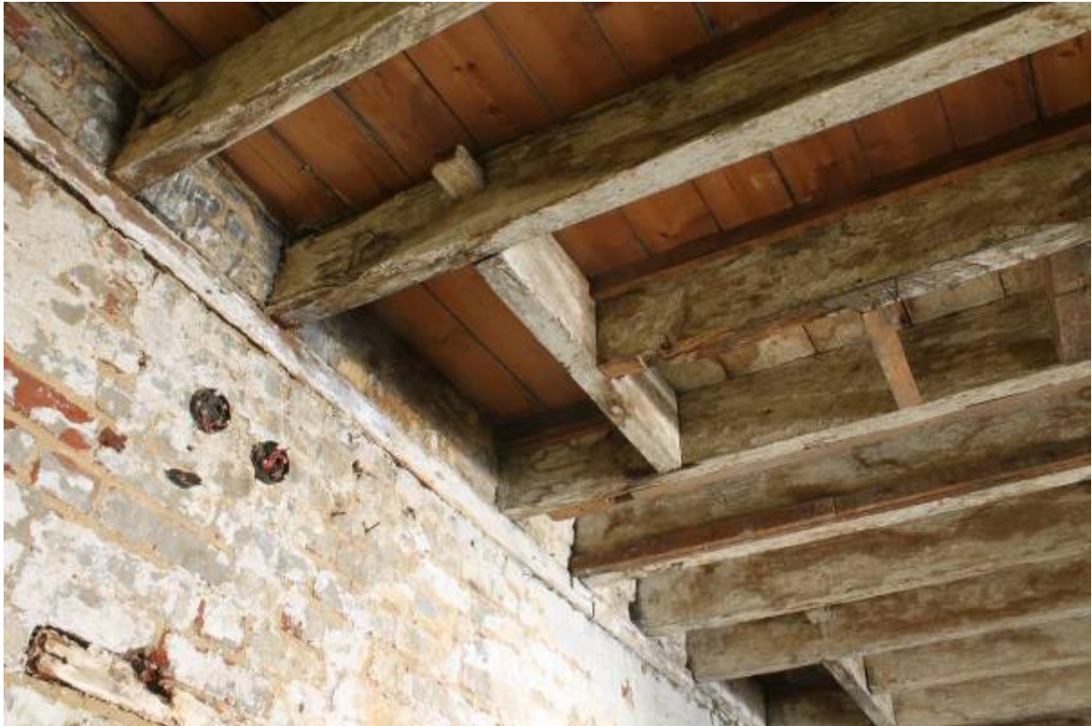
Plate 25 Detail of hatches along south wall, looking south-west and change in boarding
