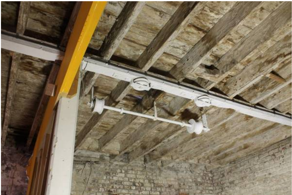
Plate 28 Section of line shafting/pulley mechanism in CG7, looking south-west
