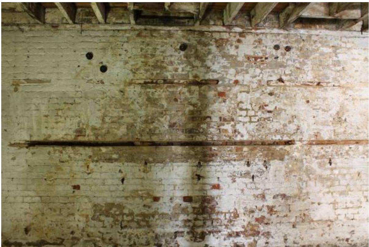
Plate 24 South wall in area CG7 (Stable C) showing mountings (battens) for former hay baskets and timber bearer (below), looking south
