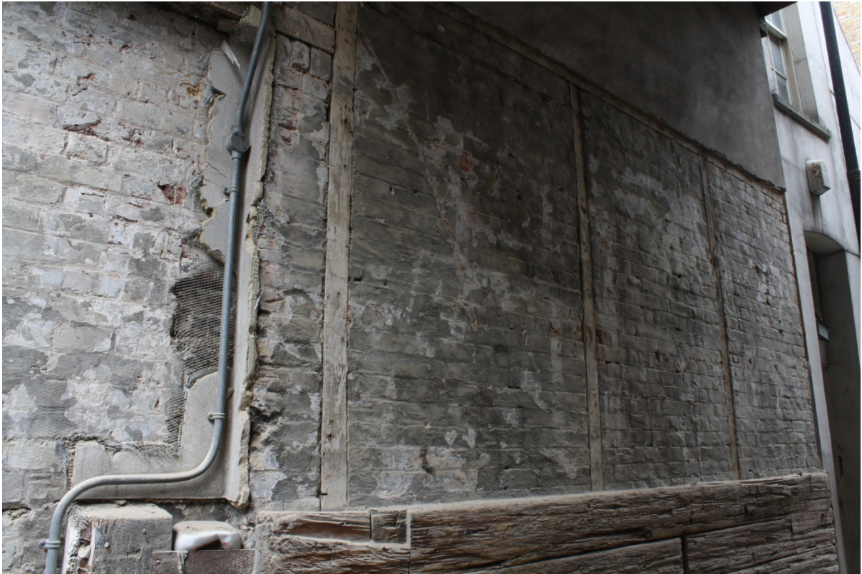
Plate 3: Upper part of the south elevation of no. 127 Borough High Street following the removal of the cement render, looking north-east
