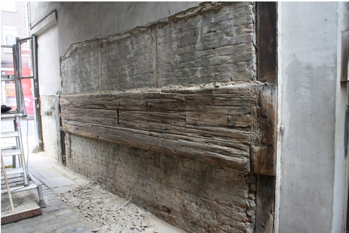
Plate 7: Large horizontal timber used to protect the south elevation of no. 127 Borough High Street from vehicle damage, looking north-west
