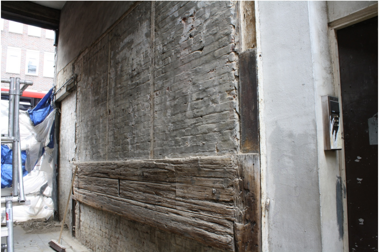
Plate 1: South elevation of no. 127 Borough High Street following the removal of cement render, looking north-west
