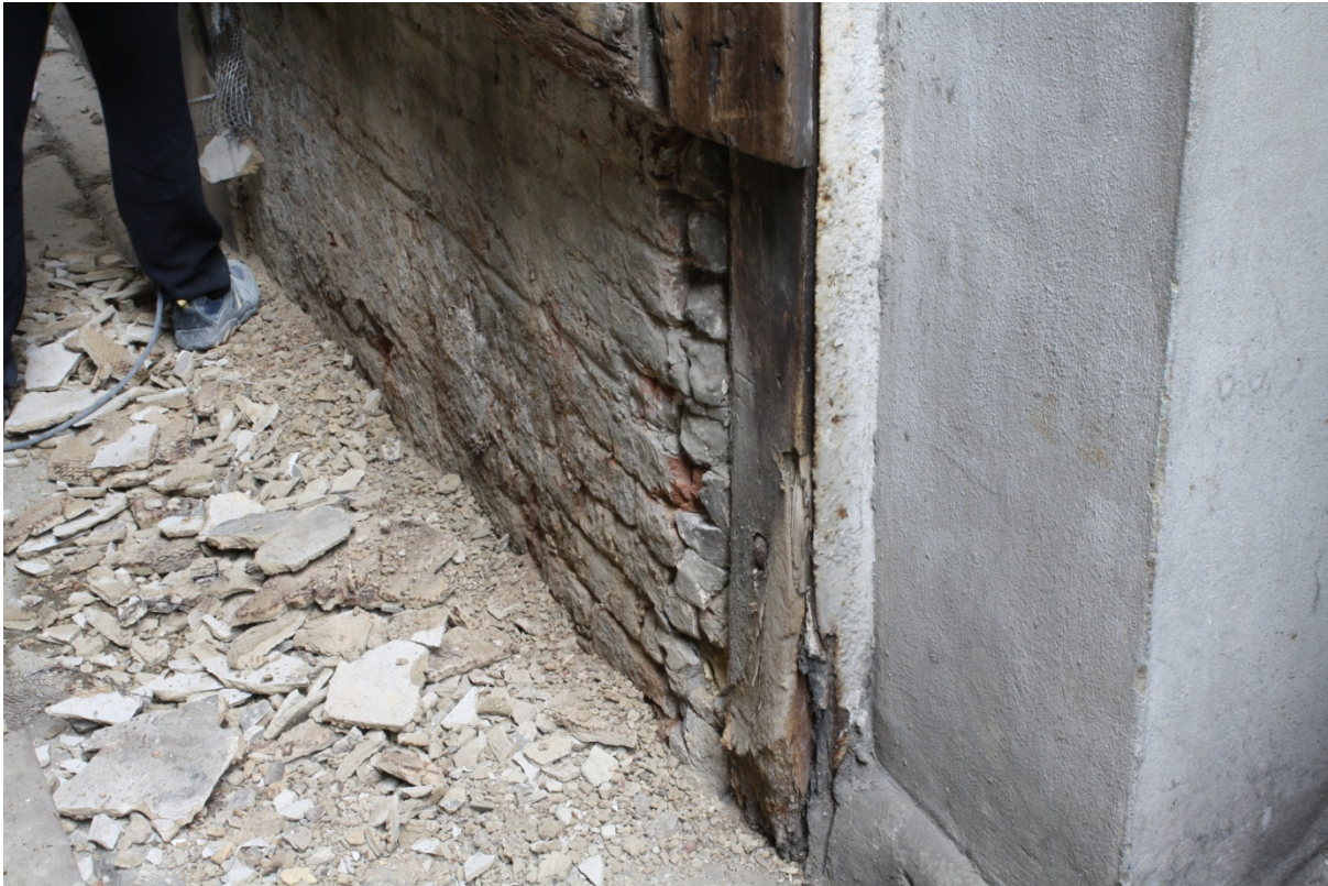
Plate 8: Timber set within RSJ at the east end of the south elevation of no. 127 Borough High Street, looking north-west
