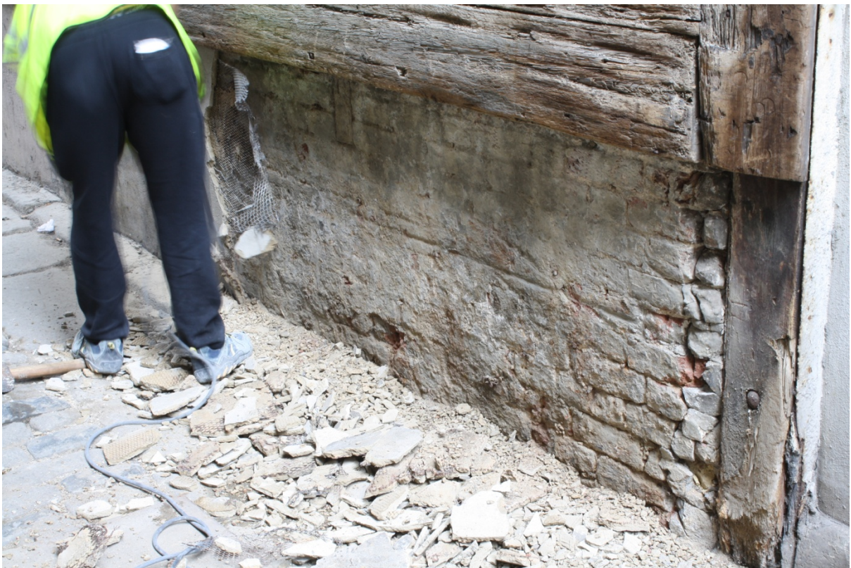
Plate 2: Lower part of the south elevation of no. 127 Borough High Street during the removal of the cement render, looking north-west
