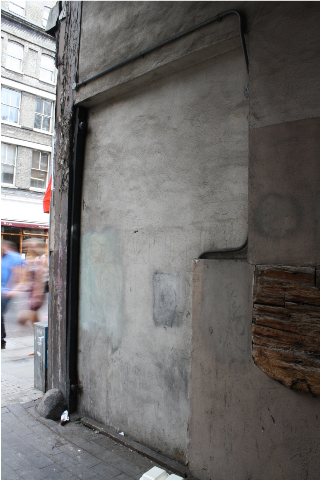
Plate 5: Recess at the west end of the south elevation of no. 127 Borough High Street before the removal of the cement render, looking north-west.
