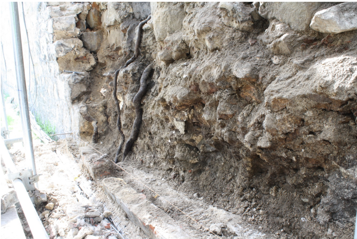
Plate 6: Tree roots observed once the outer face of the South Moat Wall had been dismantled, looking east
