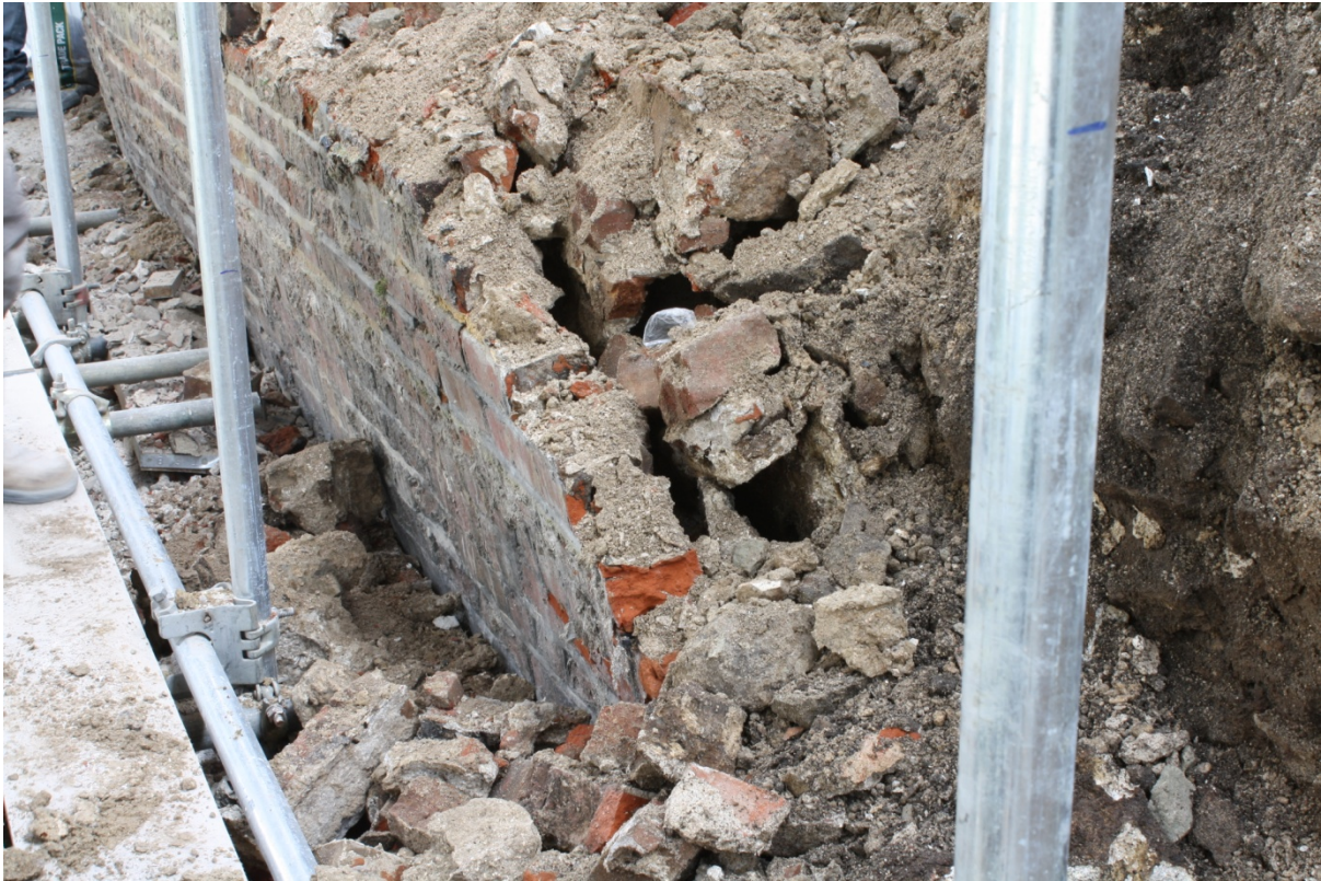
Plate 5: Lean of the brickwork in the recorded South Moat Wall, looking east
