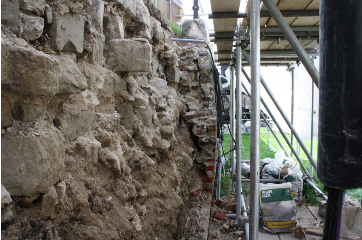
Plate 4: Bowing of the South Moat Wall at the west end of the recorded length, looking west
