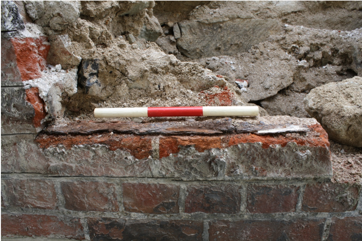
Plate 3: Hoop iron in a mortar joint within the brickwork of the outer north elevation found during dismantling, looking south
