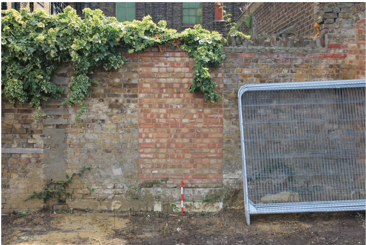
Plate 14 Wall C showing blocked door opening (northern) and red brick string courses, looking east
