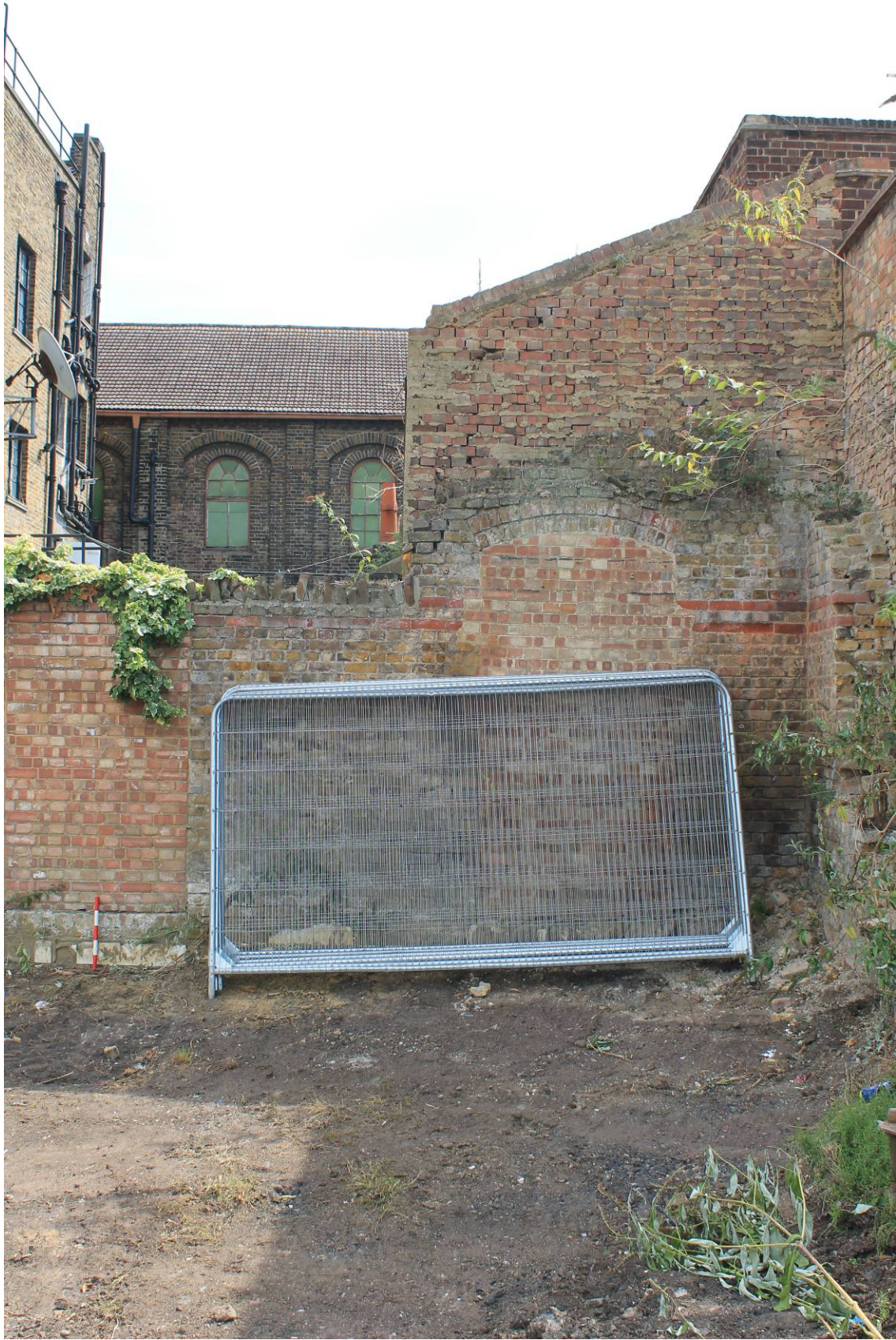
Plate 15 Wall C blocked arch headed door opening (southern) and red brick string courses, looking east
