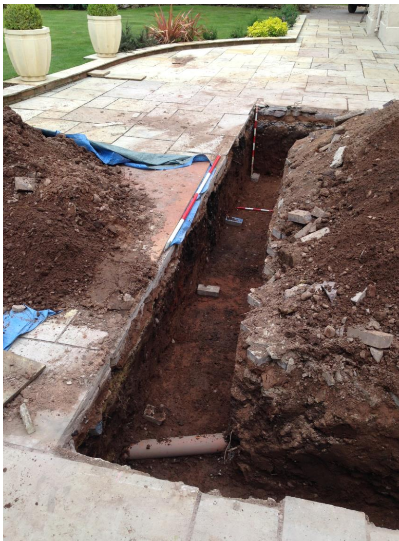
Plate 3: General shot of the east arm of the foundation trench looking south
