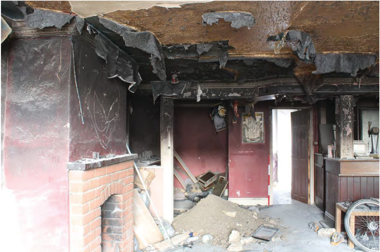
Plate 11 Area of fire damage in Bar Area (G1)
