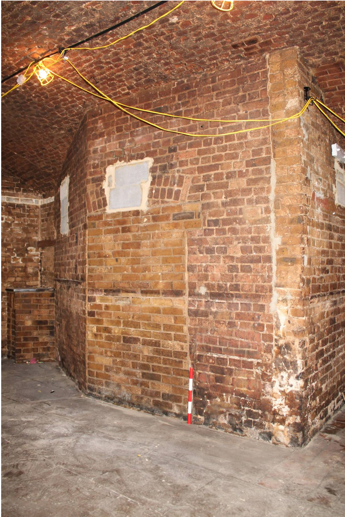
Plate 15 Canted wall and blocked former opening to vaulted areas 3 and 4, looking south.
