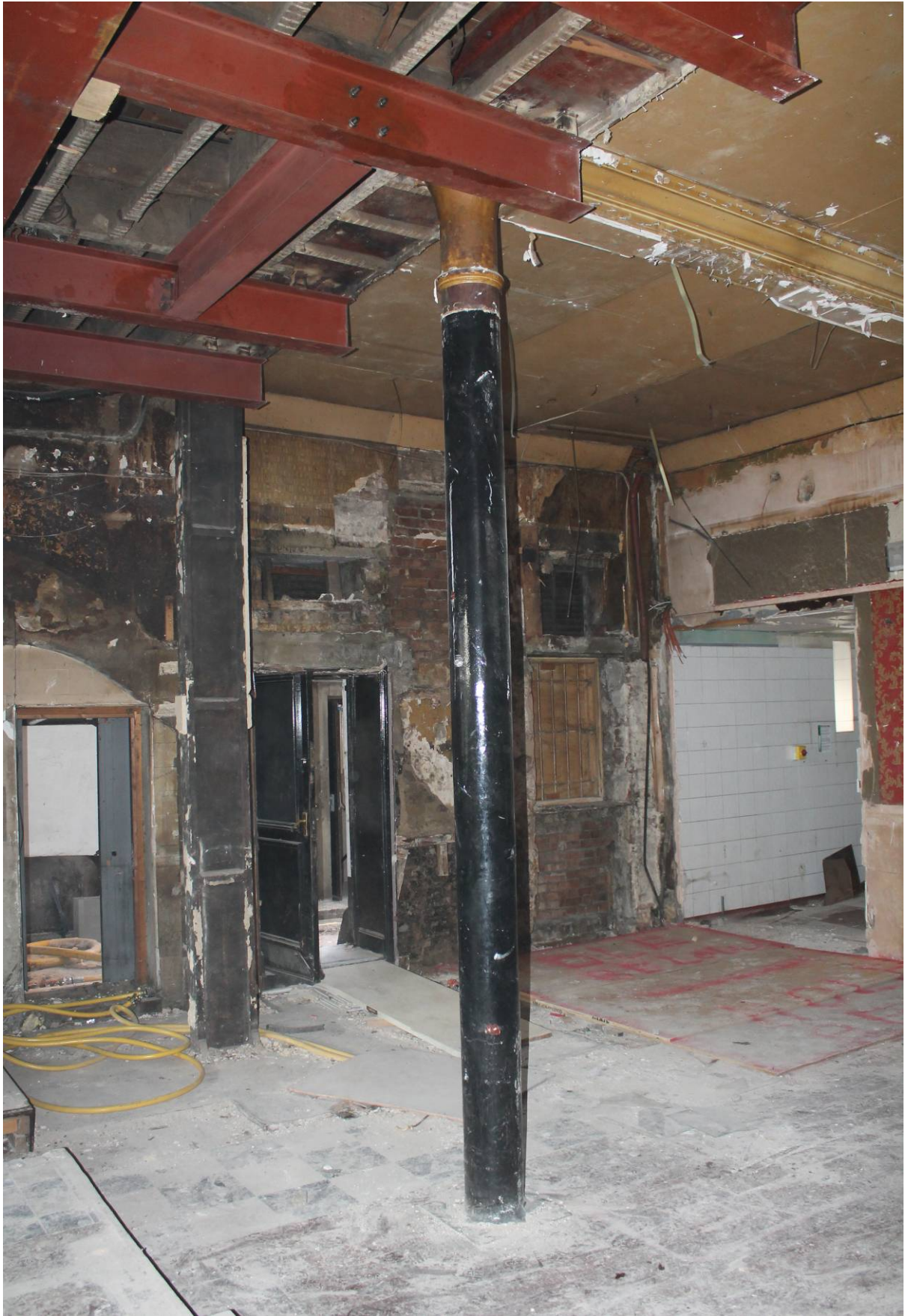
Plate 35 Cast-iron column and later stanchion, within the main bar area, looking south-west
