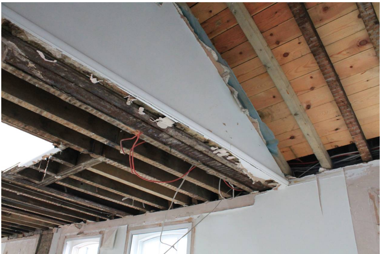
Plate 43 Junction of older range (east; left) showing floor structure to attic level, RSJ reinforcements and roof of later extension (right), looking south-east
