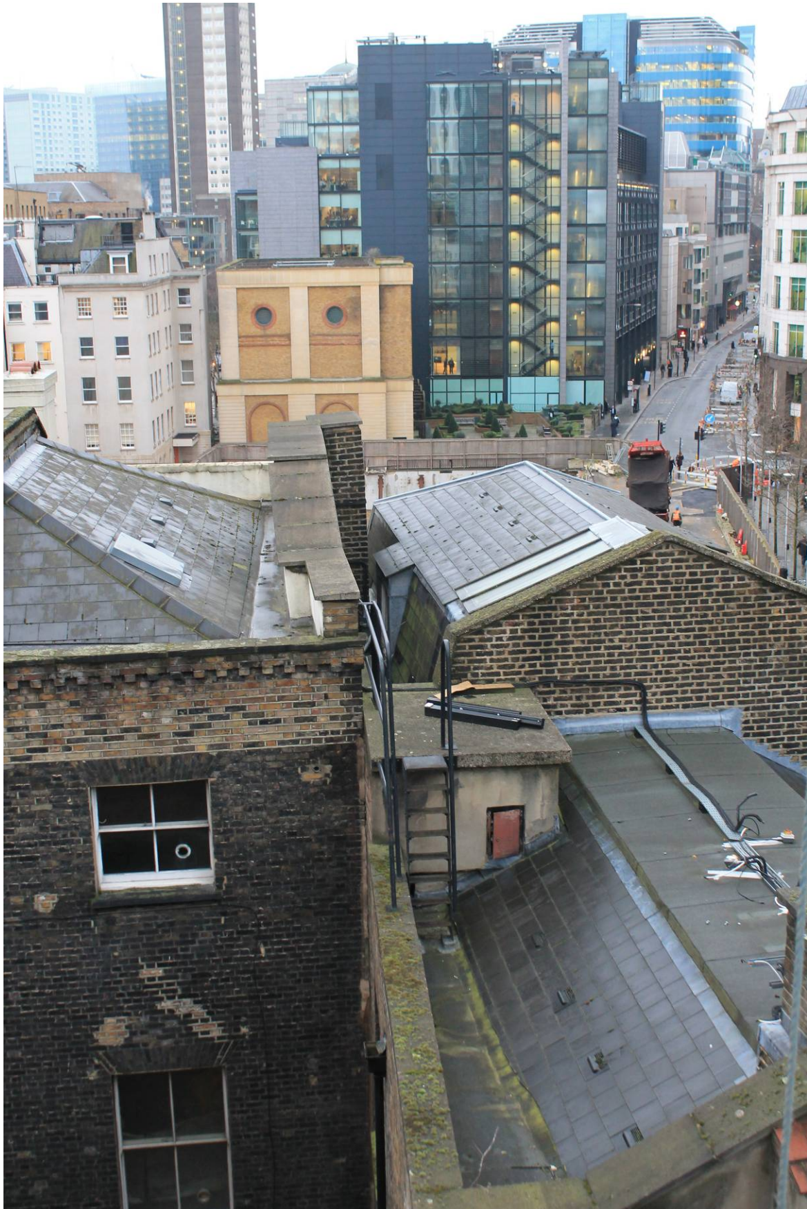
Plate 36 Rear (west) side of Mansard Roof over No. 117 Bishopsgate (right) with the lower platform roof of the extension (foreground) and hipped roof over No.119 to the north (left), looking east.
