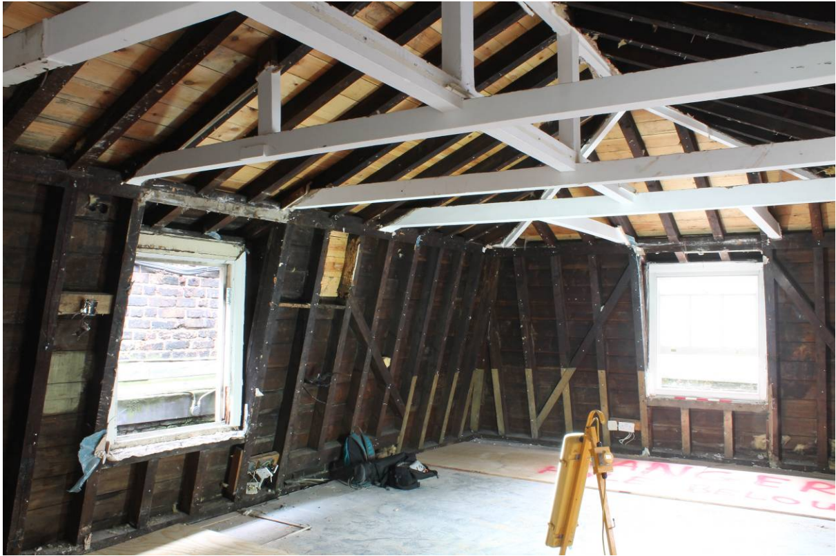
Plate 37 Primary braced Mansard Roof over the eastern part of No. 117, looking north-east
