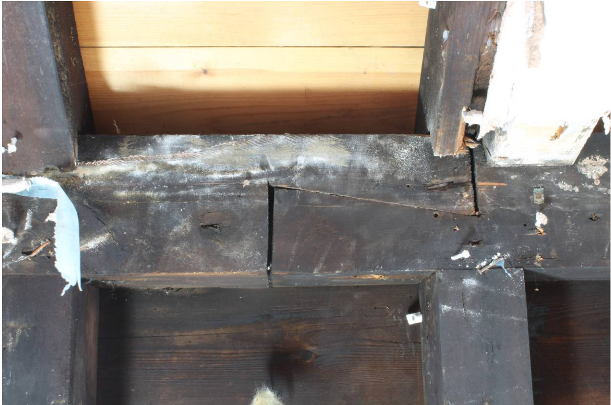
Plate 40 Edge-halved unpegged scarf joint in top rail of Mansard, looking south
