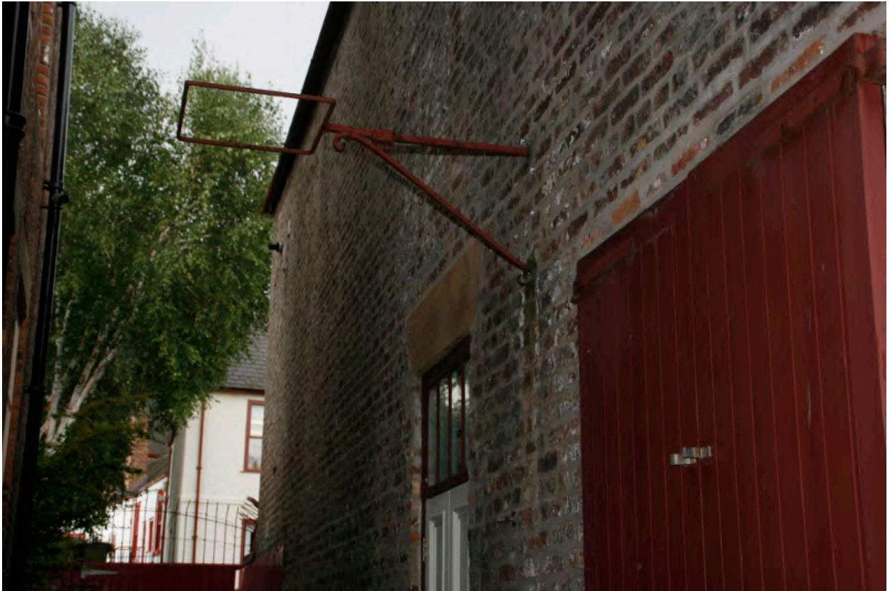
Plate 23: Centre of the rear (west) elevation of the almshouses, looking north (TRC14 BHD100 (67))
