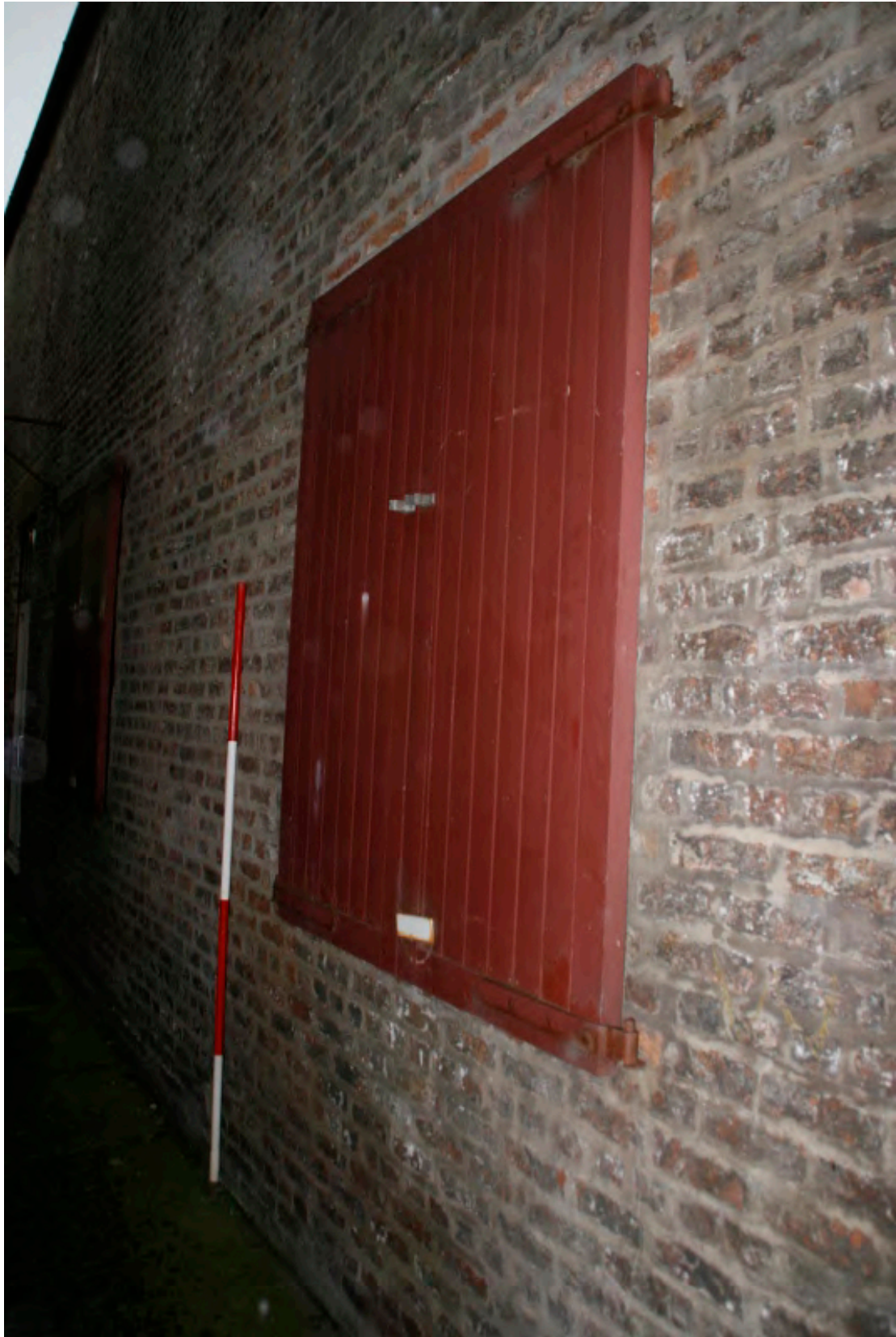
Plate 22: Inserted window with shutters at the south end of the rear (west) elevation of the almshouses, looking north (TRC14 BHD100 (66))
