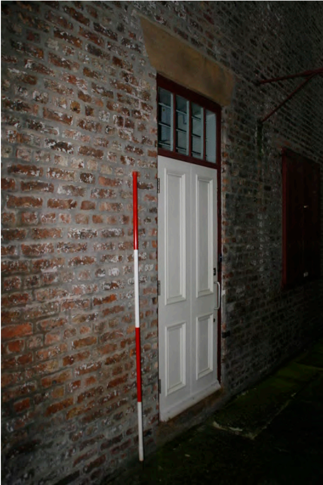
Plate 24: Inserted door with fanlight at the centre of the rear (west) elevation of the almshouses, looking south-east (TRC14 BHD100 (64))
