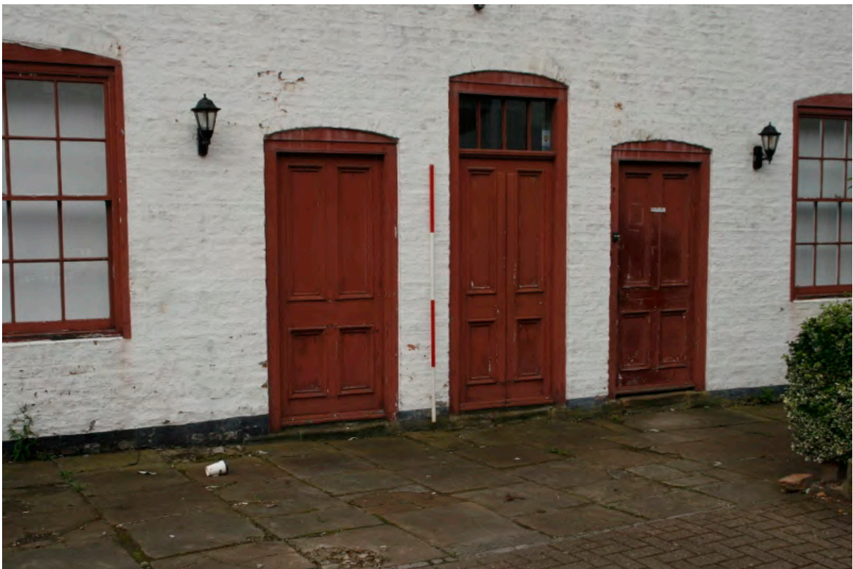
Plate 13: Three central ground floor doorways in front (east) elevation of the almshouses, looking west (TRC14 BHD100 (15))
