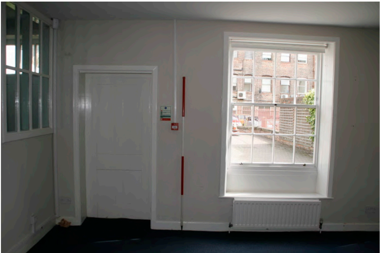
Plate 35: North end of east wall of room AHG3, looking north-east (TRC14 BHD100 (31))
