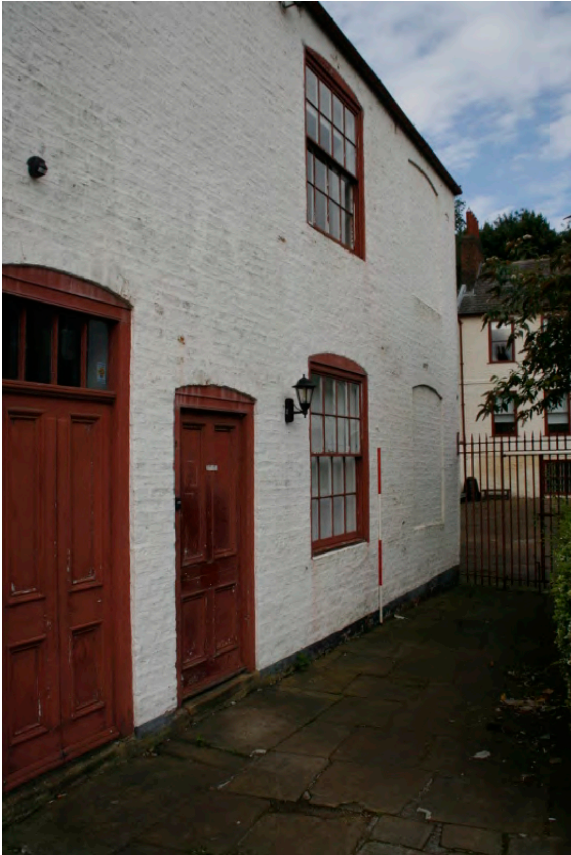
Plate 15: North end of the front (east) elevation of the Almshouses, looking north-west (TRC14 BHD100 (19))
