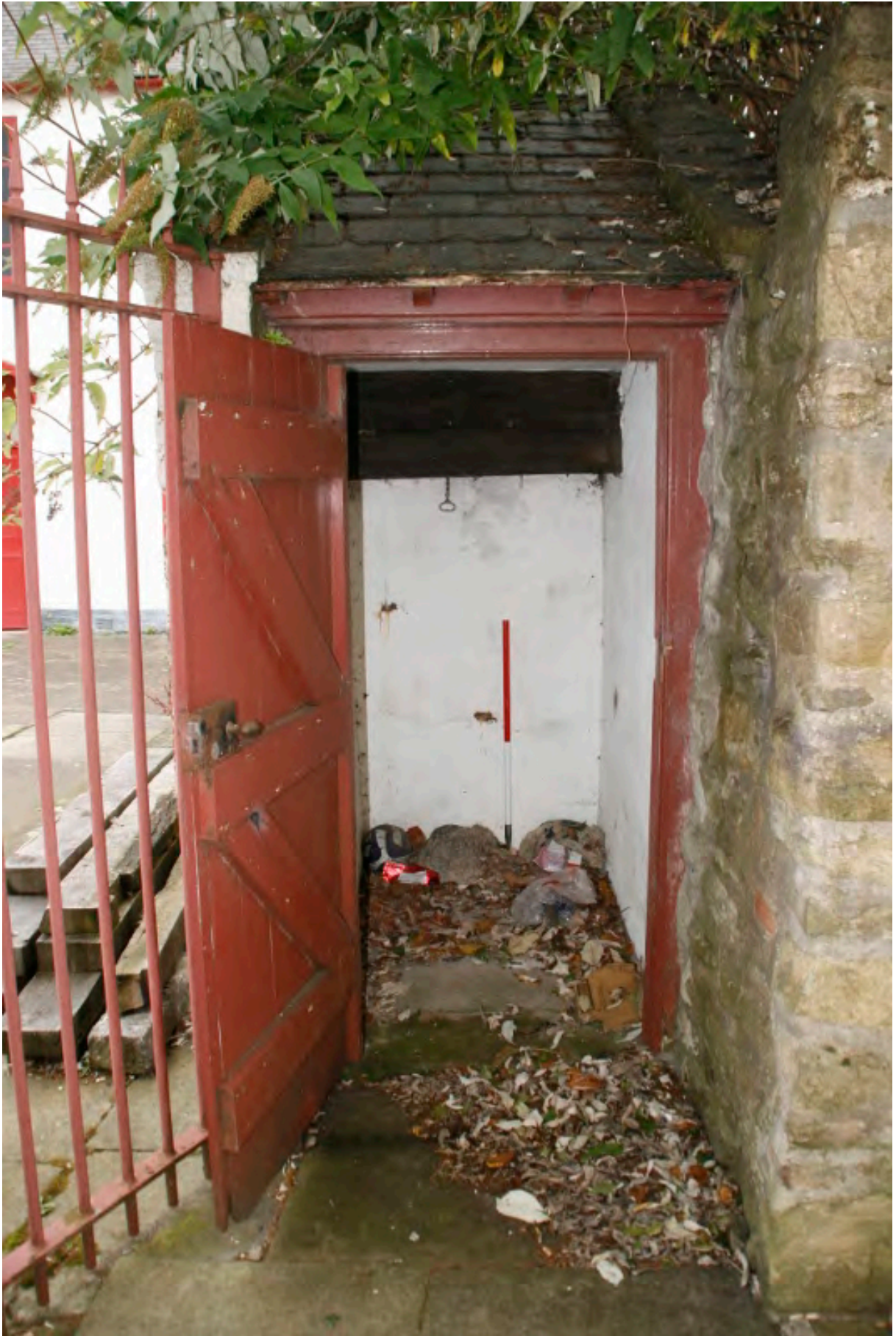
Plate 10: Interior of outside toilet at west end, looking east (PCA Ref: TRC14 BHD100 (09))
