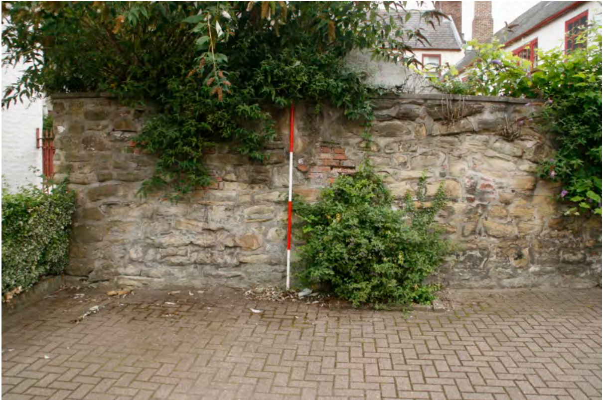
Plate 5: Red brick repair to stone wall, looking north (PCA Ref: TRC14 BHD100 (04))
