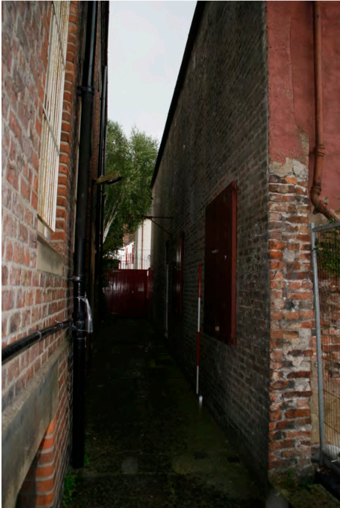
Plate 21: South end of the rear (west) elevation of the Almshouses, looking north (TRC14 BHD100 (65))
