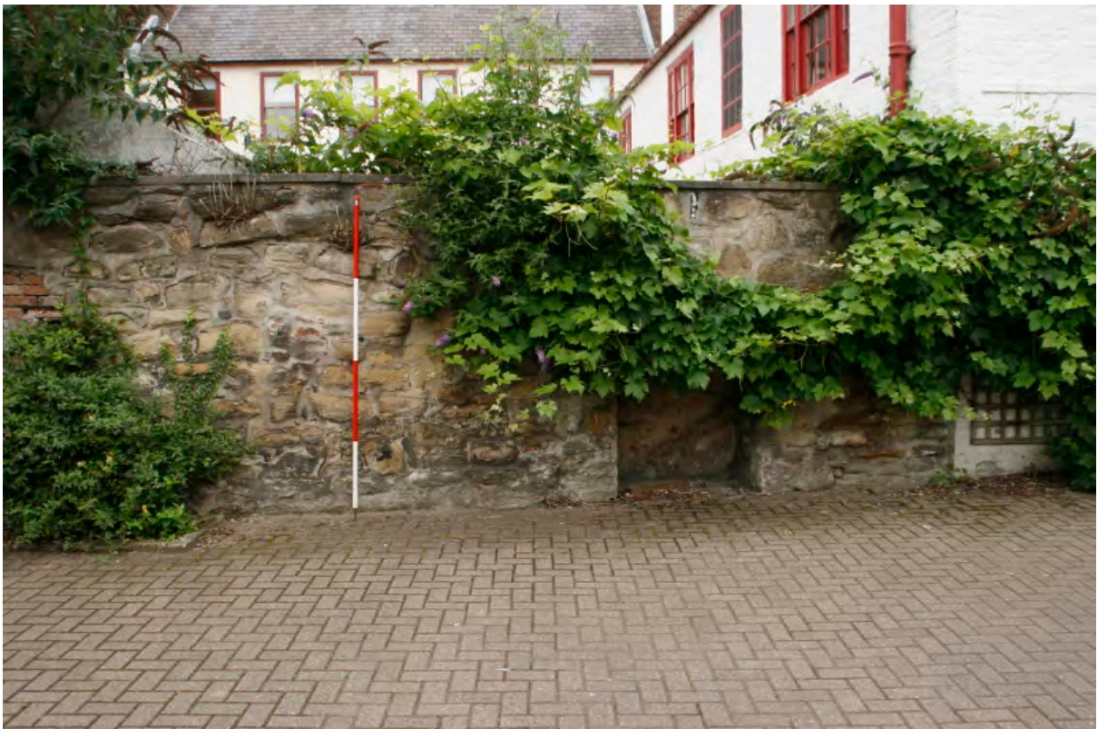
Plate 6: Blocked opening towards the west end of the stone wall, looking north (PCA Ref: TRC14 BHD100 (05))
