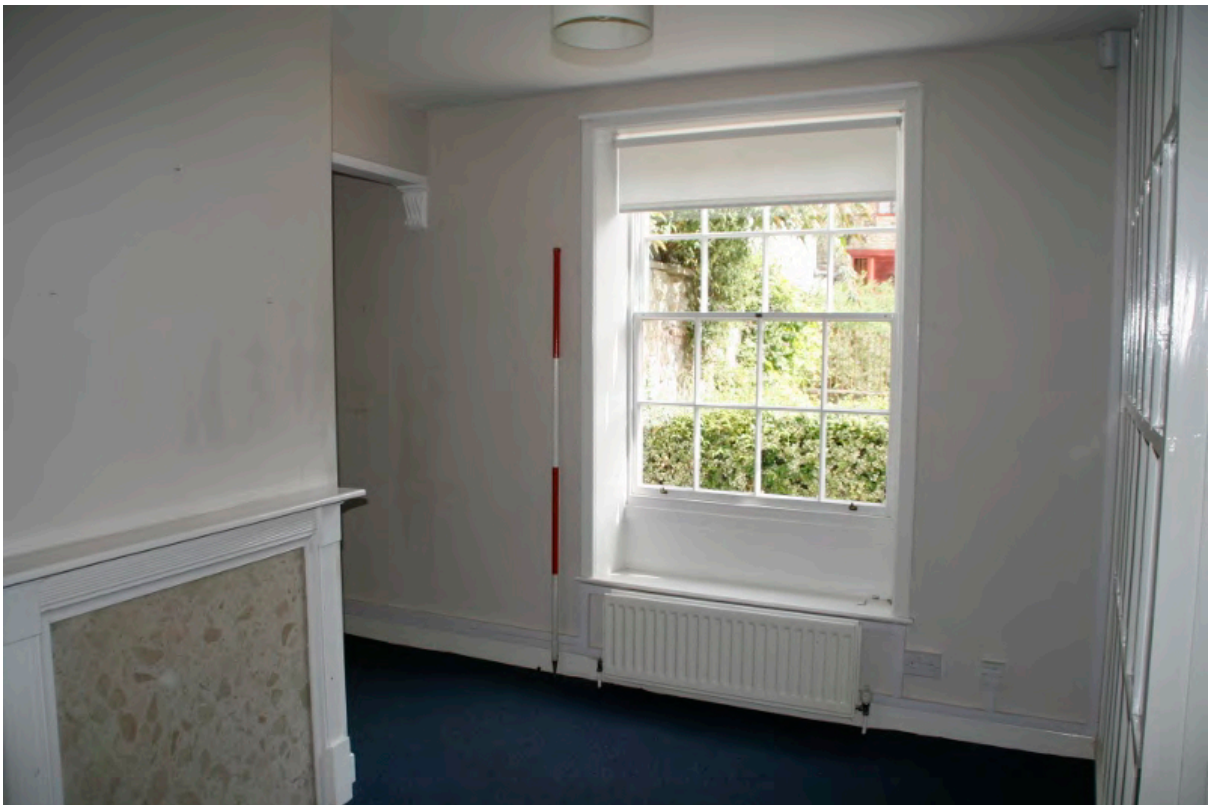
Plate 30: Sash window in east wall of room AHG2, looking east (TRC14 BHD100 (38))
