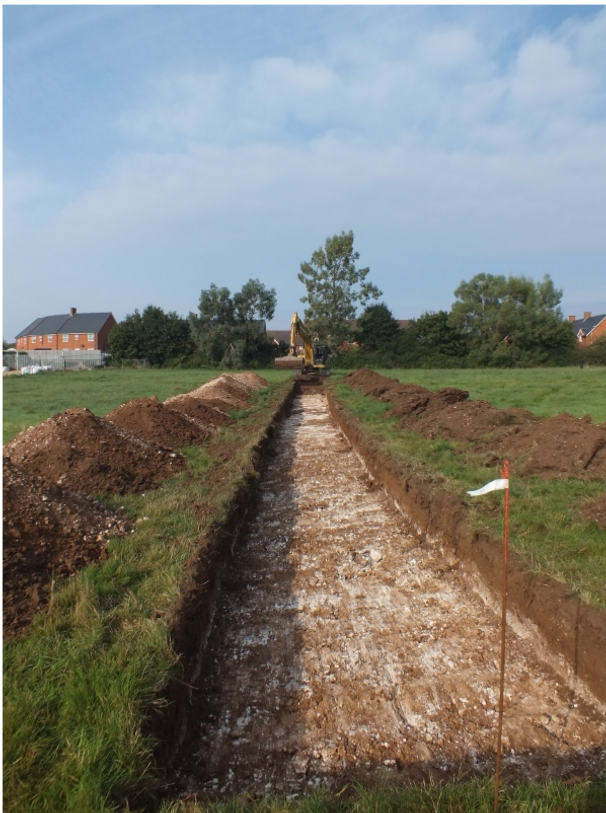
Plate 1: Working shot of Trench 1 being dug with 360° digger, looking west (WGGL14 D1 (2))
