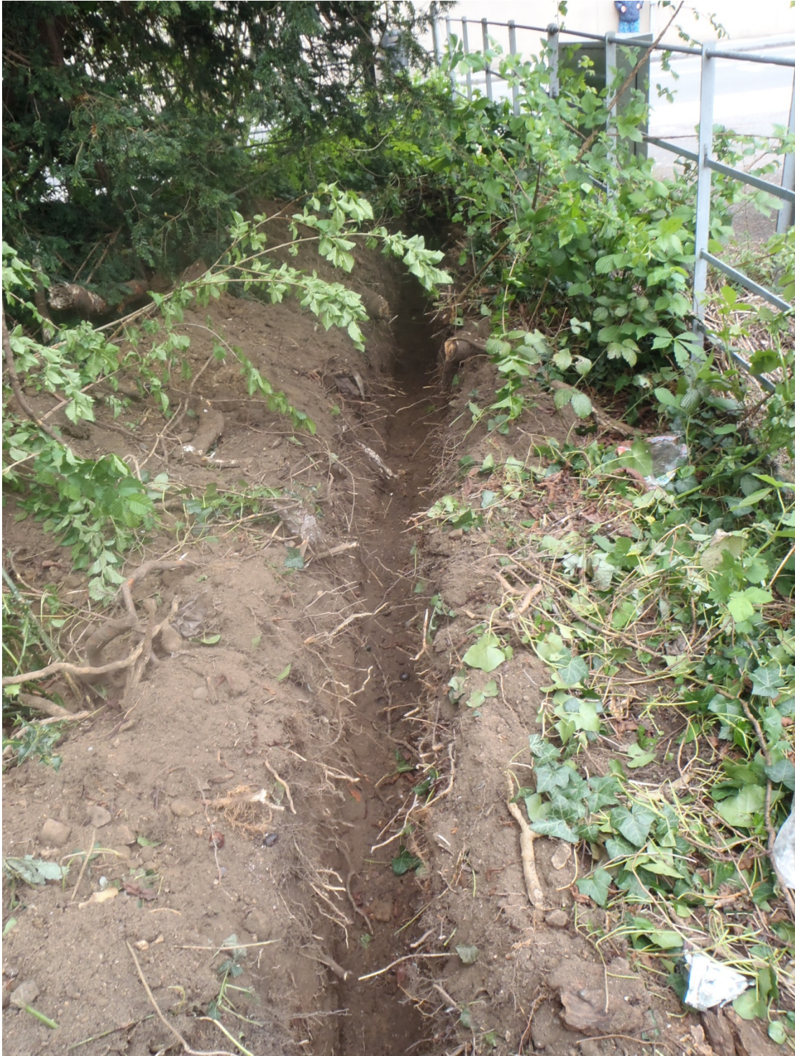
Plate 3: Telecommunications trench, looking northeast across area of former 18 th century garden maze
