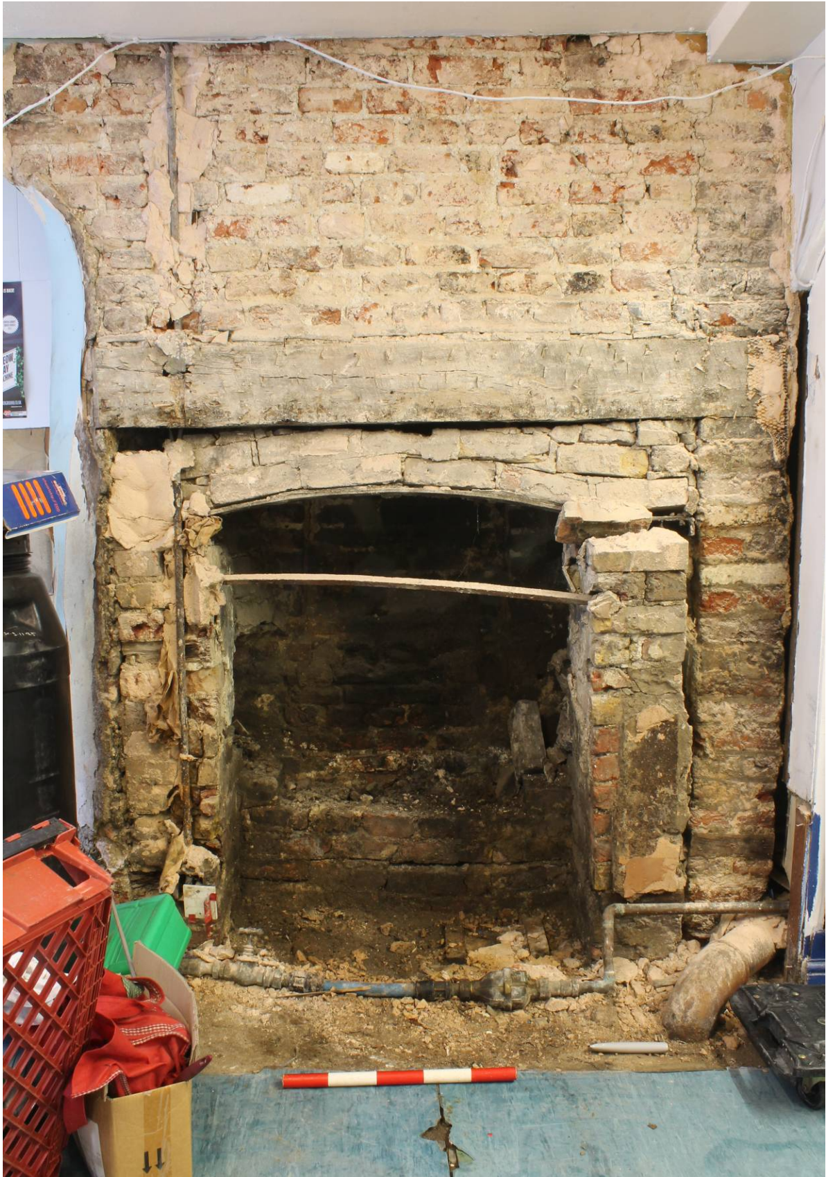
Plate 6 Fireplace with corbelled angle within front part of the building (Area 1), looking east.
