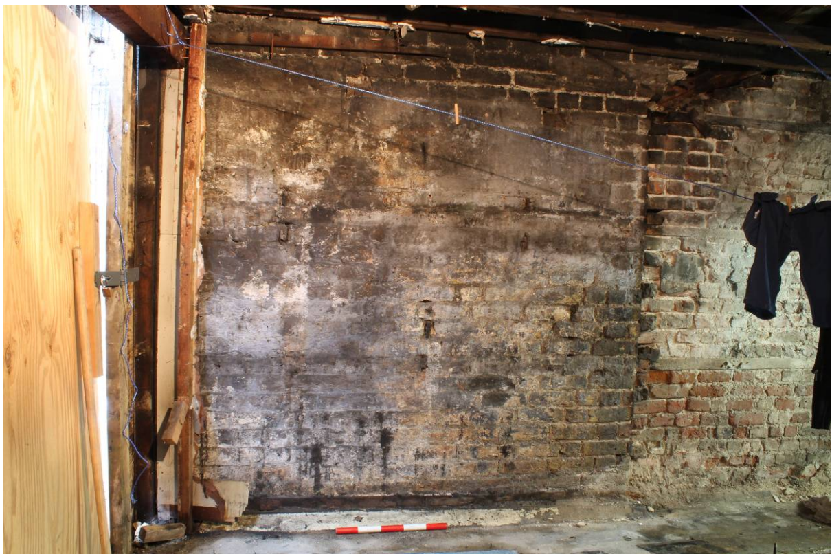
Plate 16 Flank wall of mid to late 19 th century extension to adjacent butchers (No. 31), looking west
