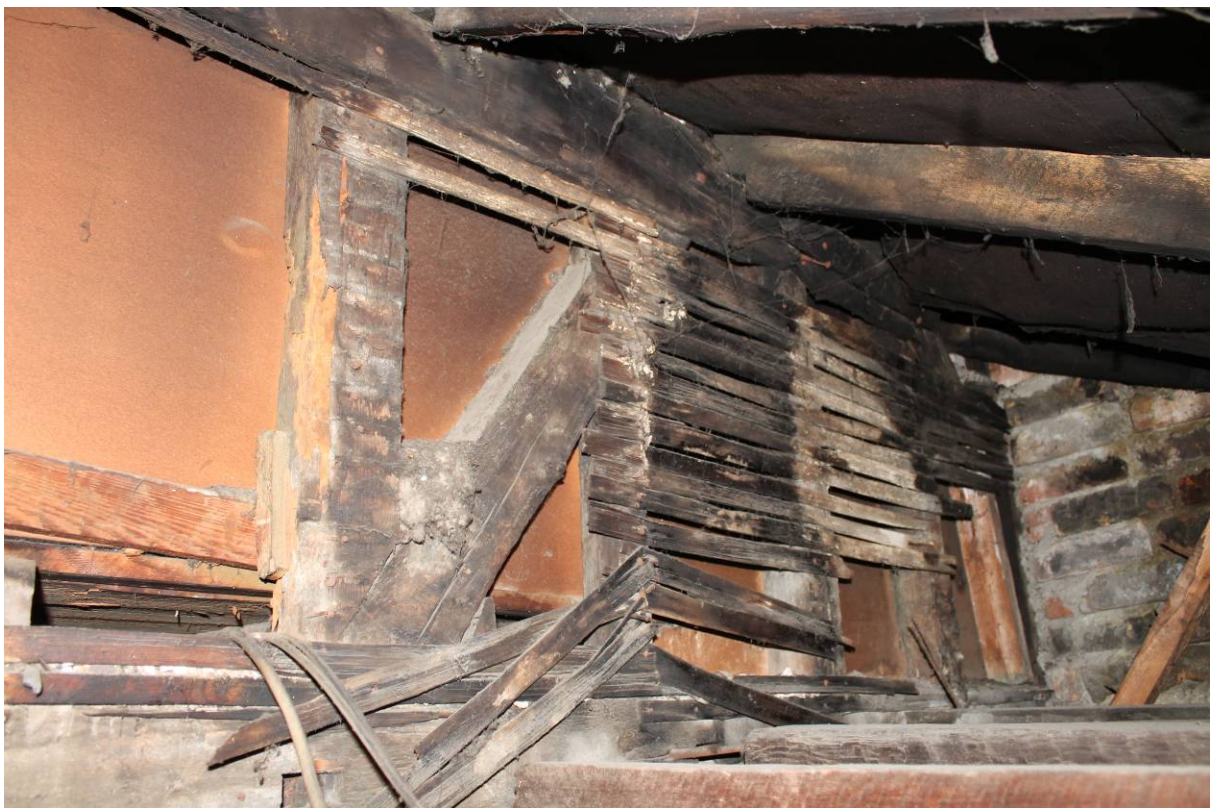
Plate 10 Primary braced upper register looking east toward No. 25, showing lathes and lean-to roof
