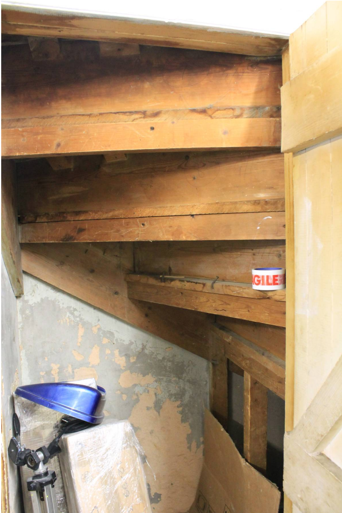
Plate 8 Under-stairs cupboard revealing the structure of the narrow winder stairs, looking east
