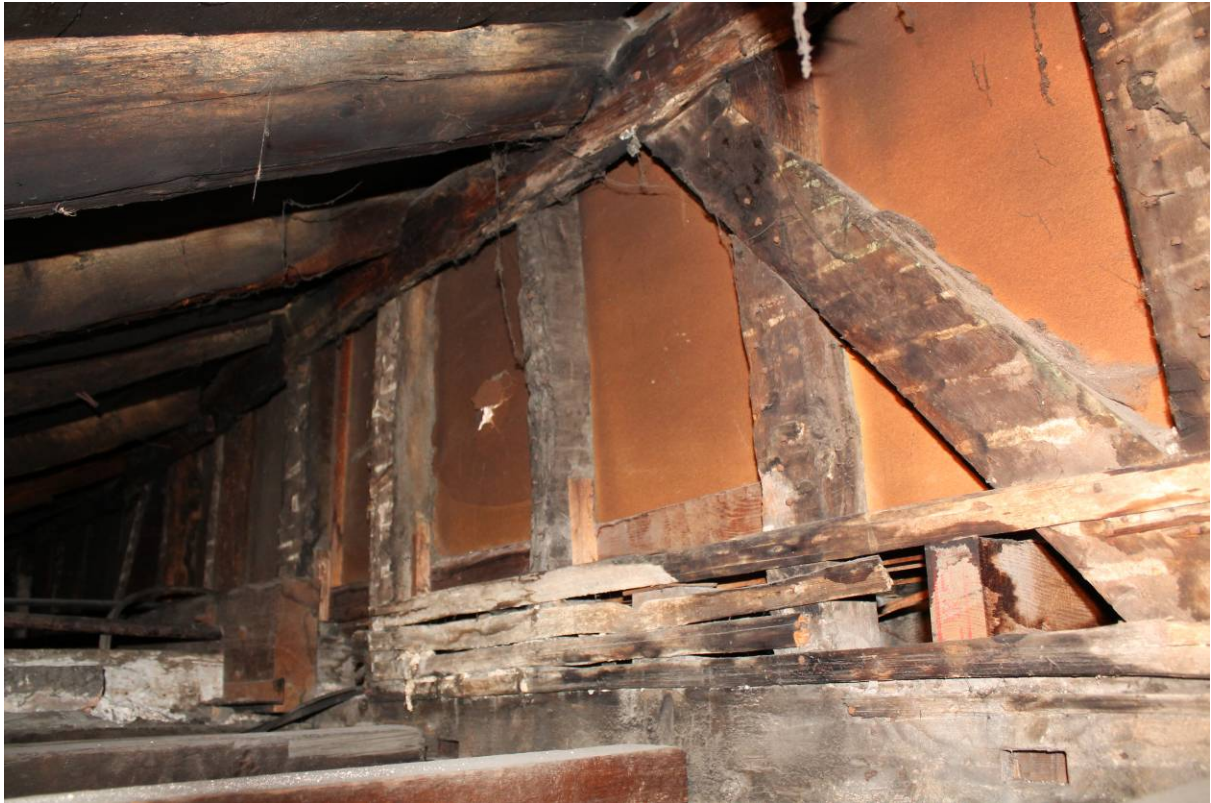
Plate 9 Primary braced upper register and mid rail, below lean-to roof, to the rear of No. 29 and 31
