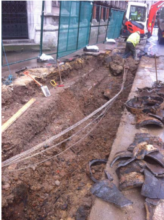
Plate 1: Most of the trenches were comprised entirely of fill of modern and antiquated services. This photo shows excavation underway in Trench 3 in the Strand, immediately to the east of the main entrance to the RCJ.
