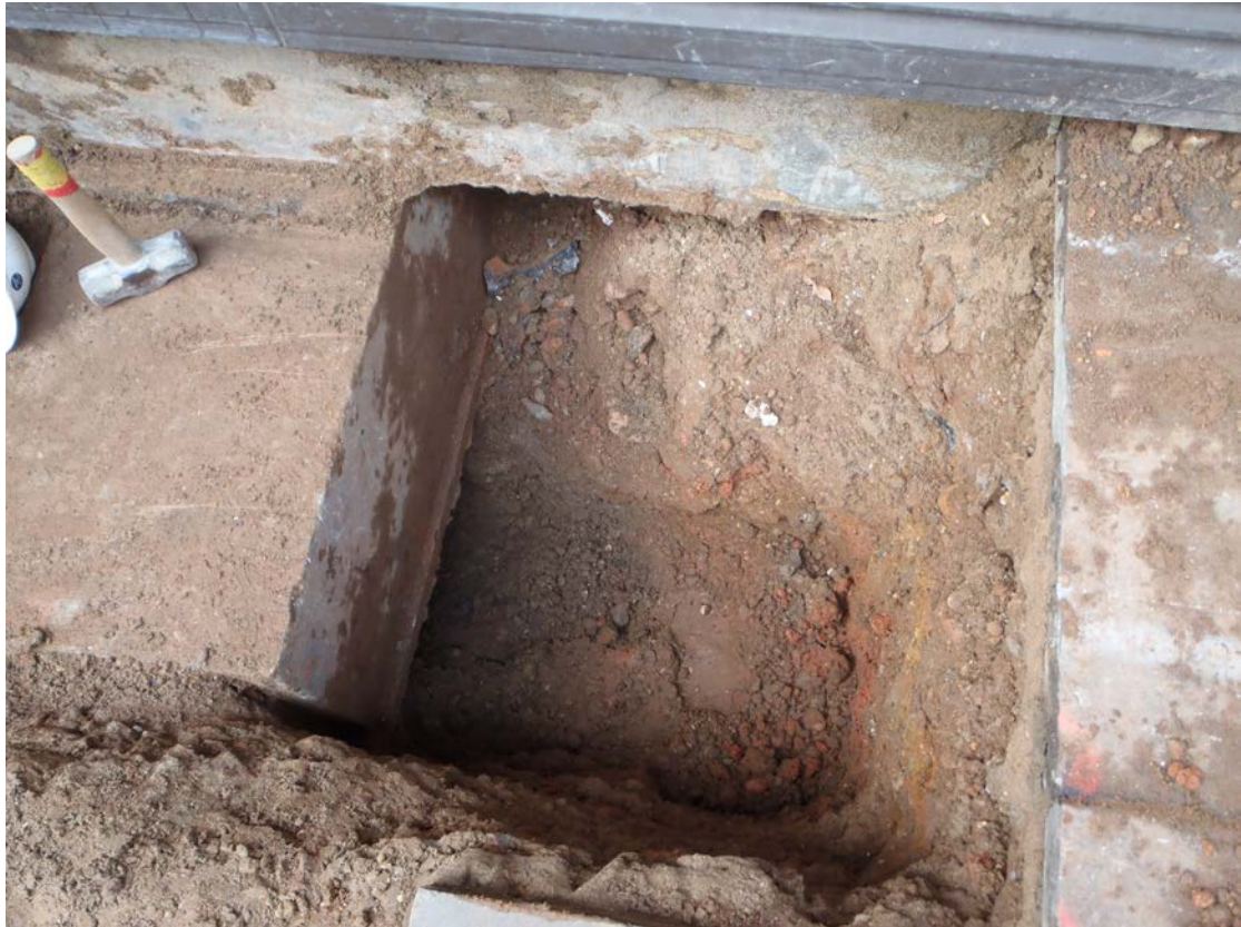
Plate 2 West facing view of Test Pit 2; showing red burnt clay [1] and pile cap
