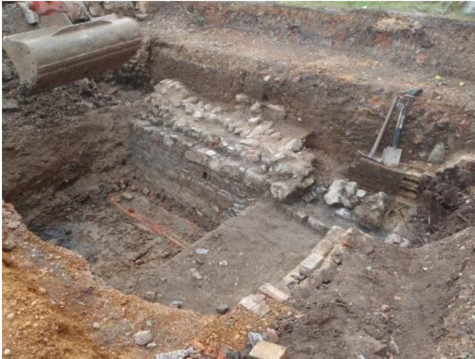
Plate 3. Trench 2 working shot, looking southwest prior to machine excavation of brick culvert flanking north-south wall 209 .
