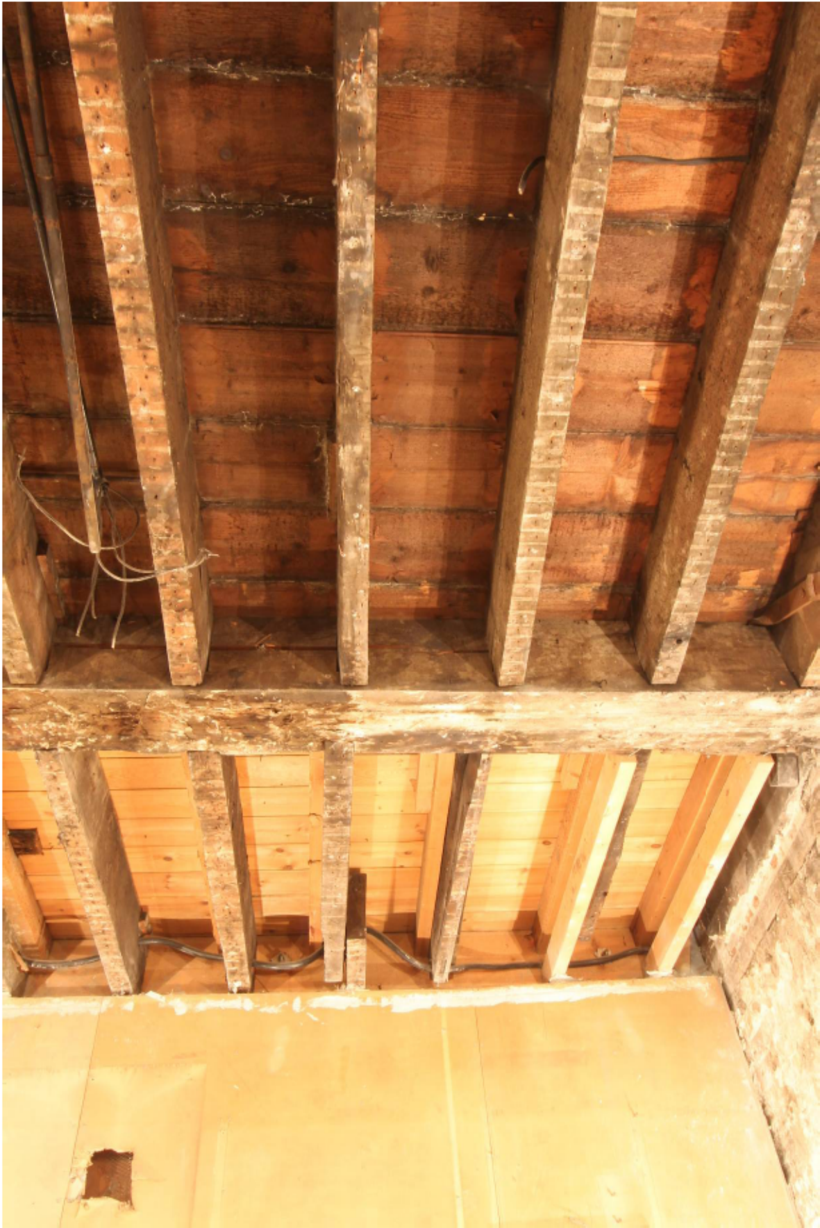
Plate 8 Heavy binding joist and common floor joists over room GF1, looking east
