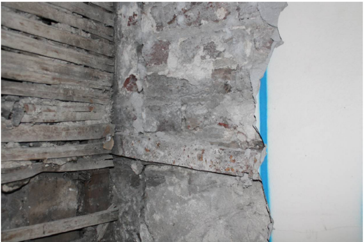
Plate 15 Straight joint and wrought iron strap in the north-west corner of sitting room FF1, looking north-west
