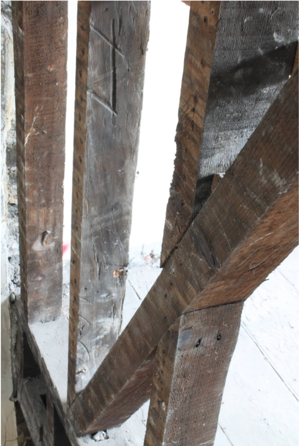
Plate 32 Baltic marks on primary bracing of stairwell TF2 (note nailing stud to tension brace), looking north-east
