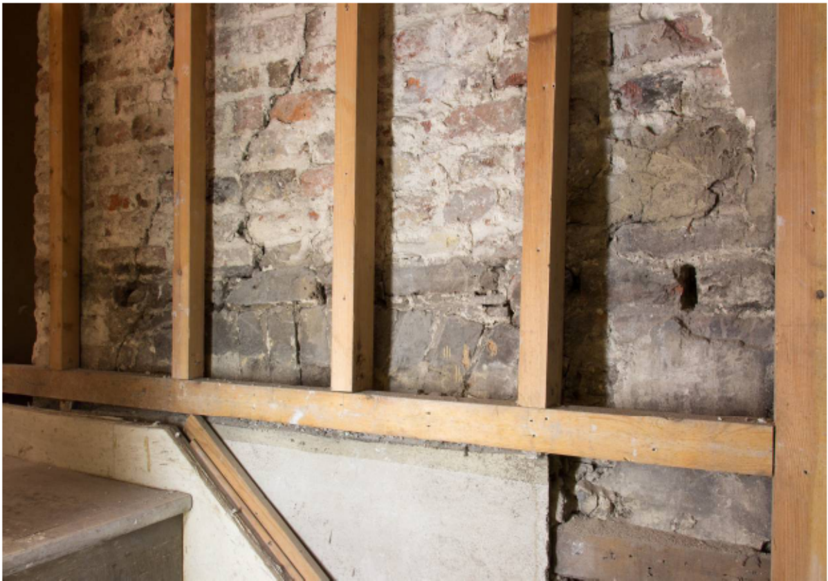
Plate 10 Segmental brick arch of fireplace covered by modern stair in GF2, looking north-west
