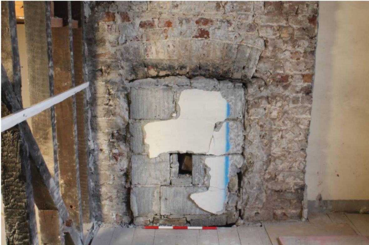
Plate 25 Blocked fireplace in the north wall of room SF3 (also shows fire damaged wall frame), looking north
