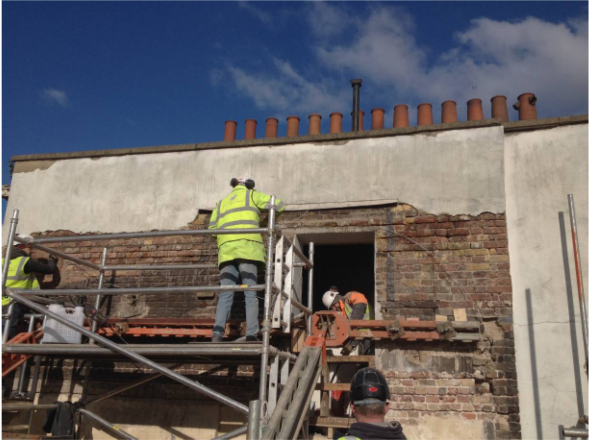
Plate 5b Southern elevation of no. 127 Borough High Street at third floor level, looking north (Photograph supplied by Michael Groves, LTS Architects)
