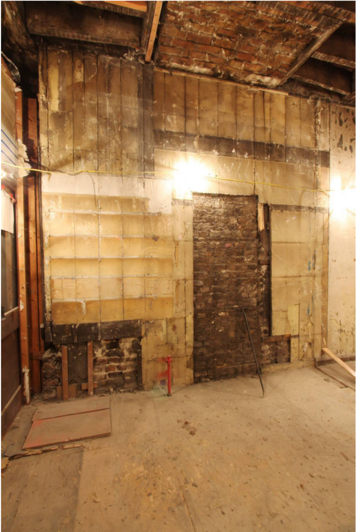
Plate 7 Former kiosk (GF1) after soft stripping out showing remains of historic barding covering the walls, looking north
