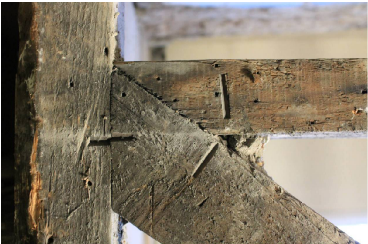
Plate 24 Original chiselled numerical assembly marks on primary braced wall frame in the east wall of room SF2, looking east
