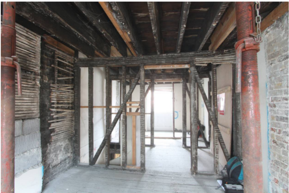
Plate 29 Room TF1 looking east towards primary braced wall frames of stairwell TF2
