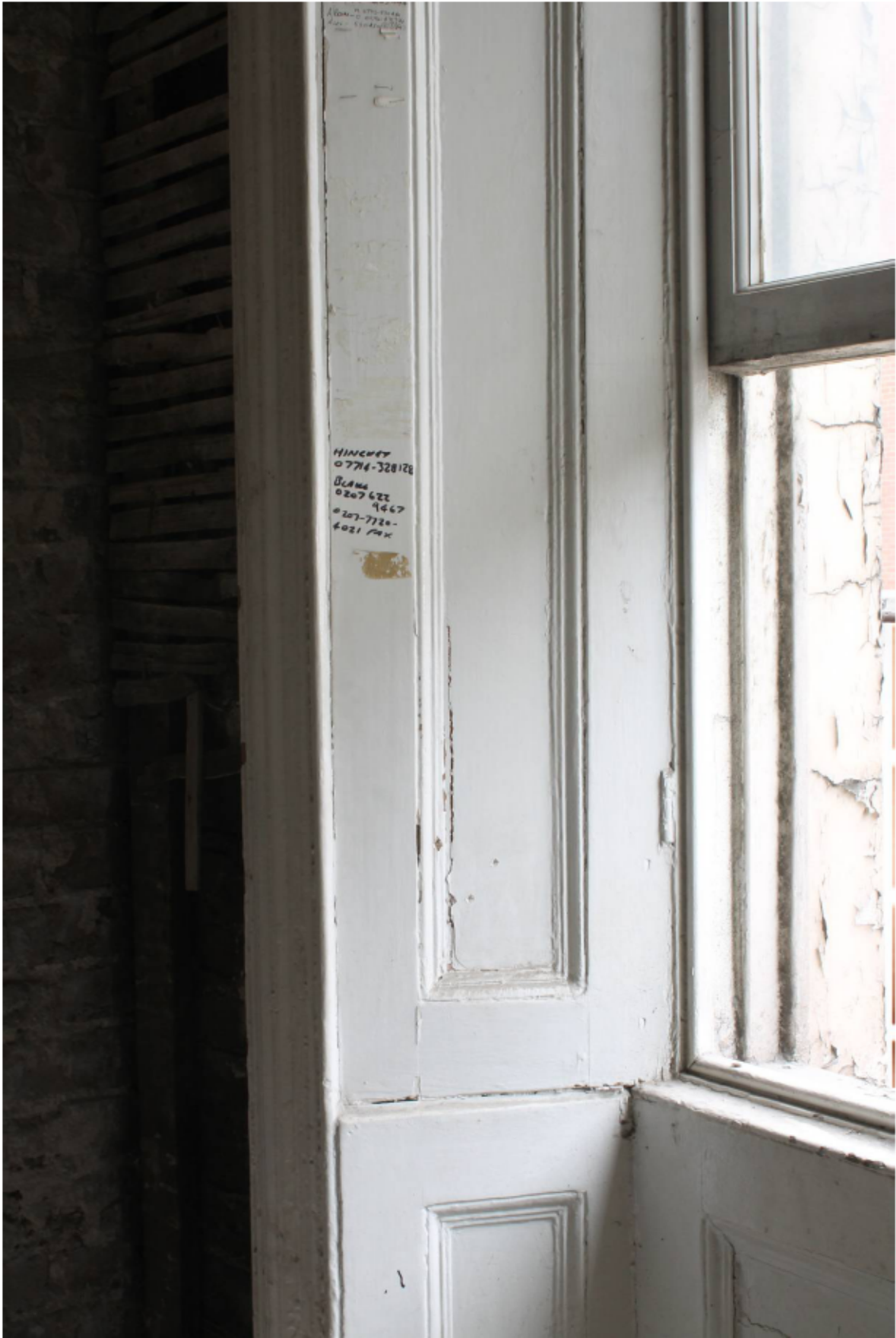
Plate 17 'Pinned back' window shutters to west window in room FF1, looking south-west
