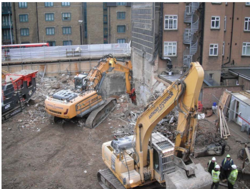
Plate 2: View northeast overlooking removal of basement slab at northeastern corner of the site. This work confirmed that the basement had truncated the site beyond the level of the natural superficial geology
