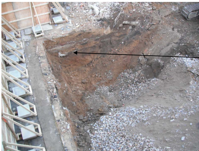
Plate 3: View north overlooking obstruction removal at central western side of the site. Note the extensive concrete foundations of the former building which extend to approximately 2.0m BGL, truncating into the surface of the natural gravels.
