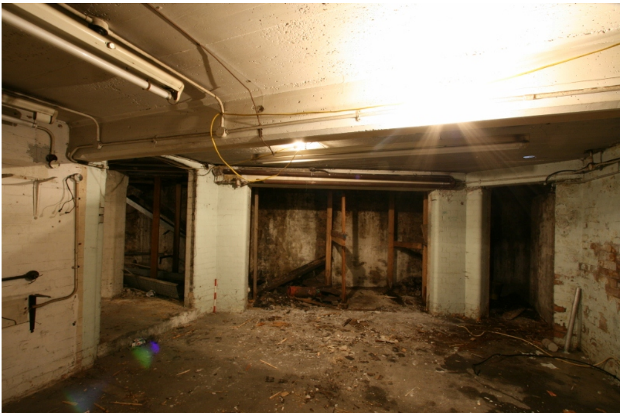
Plate 50: Basement room B2B3 showing entrances to pavement vault area, looking south (VAL14 D100 (60))
