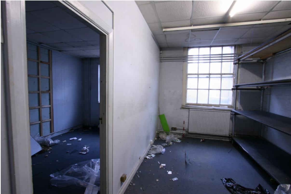
Plate 57: Ground floor rooms B2G7 (right) and B2G8 (left) created by insertion of modern partition wall, looking south-west (VAL14 D100 (35))
