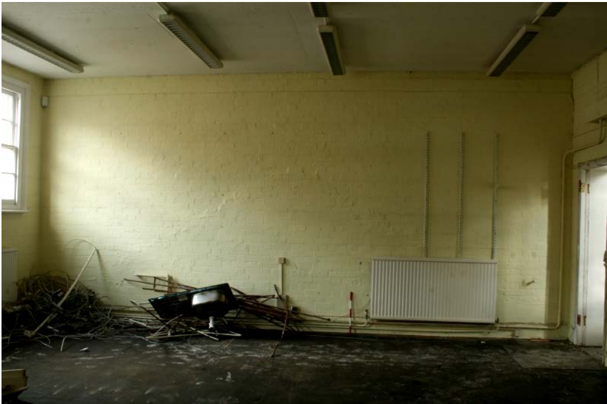
Plate 86: Scarring on north wall of second floor room B2S1, looking north (VAL14 D100 (101))
