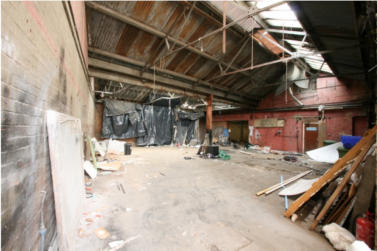
Plate 41: Steel trusses and corrugated roof covering loading/delivery area B2G2, looking south-west (VAL14 D100 (25))
