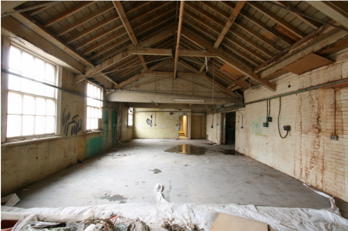
Plate 83: Original timber roof trusses in first floor room B1F1, looking north (VAL14 D100 (115))
