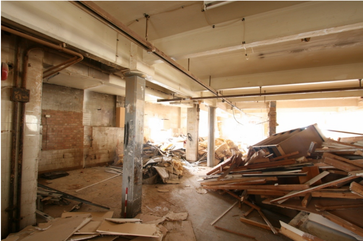
Plate 81: Cast iron columns encased in concrete and overhead beams in first floor room B2F1, looking east (VAL14 D100 (113))
