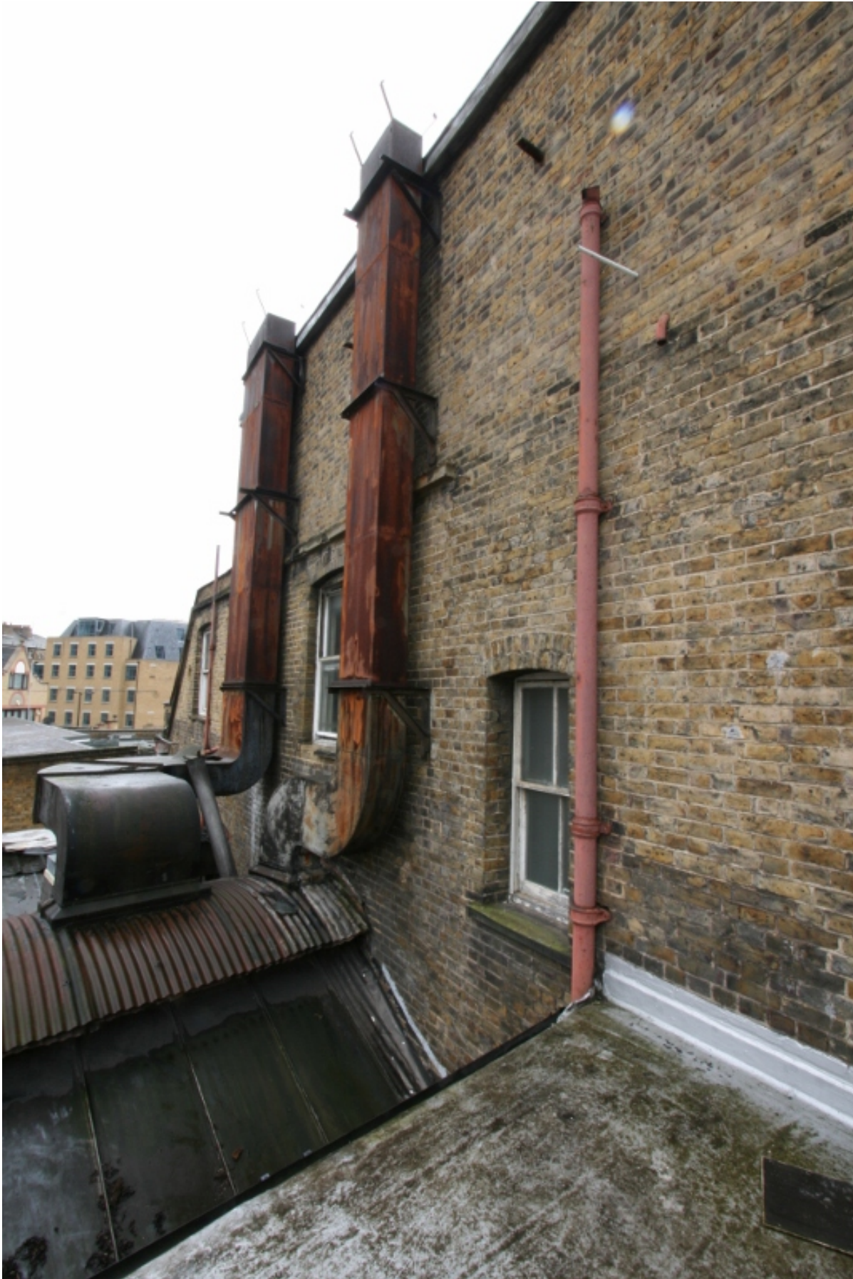
Plate 37: Second floor north elevation of nos 17-19 Valentine Place/no. 21 Webber Street, looking south (VAL14 D100 (124))
