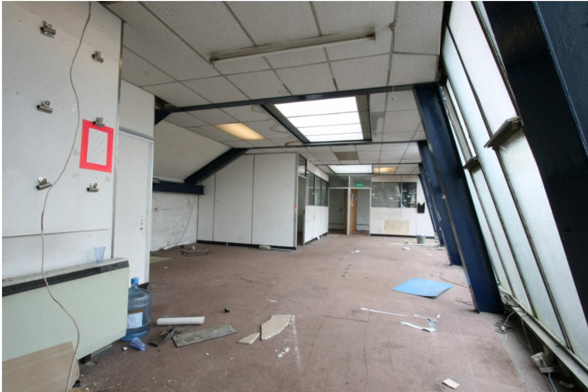
Plate 21: Small office space (B1F1) on first floor of nos 3-5 Valentine Place, looking south (VAL14 D100 (134))
