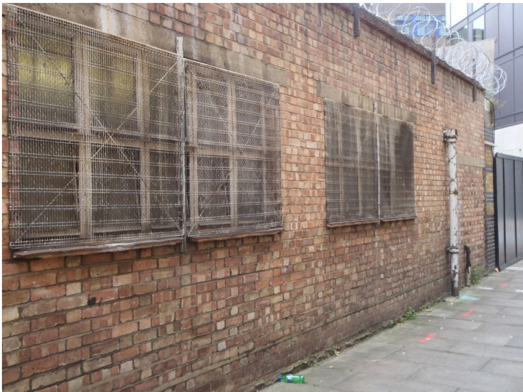
Plate 10: Detail showing northern end of nos 3-5 Valentine Place rear (east) elevation fronting onto Valentine Row, looking north-west
