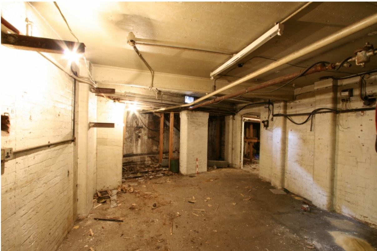
Plate 48: Basement room B2B2 showing entrance in pavement vault area, looking south-west (VAL14 D100 (55))
