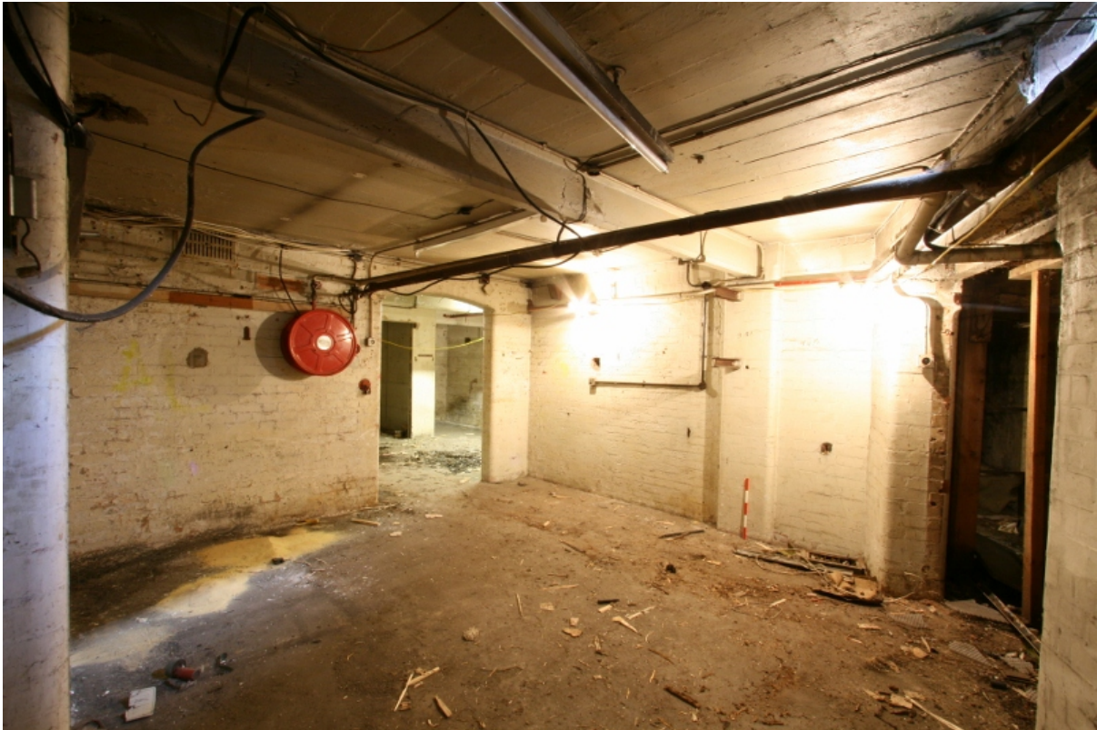
Plate 47: Basement room B2B2 showing entrance into B2B1 (left) and pavement vault area (right), looking north-east (VAL14 D100 (56))
