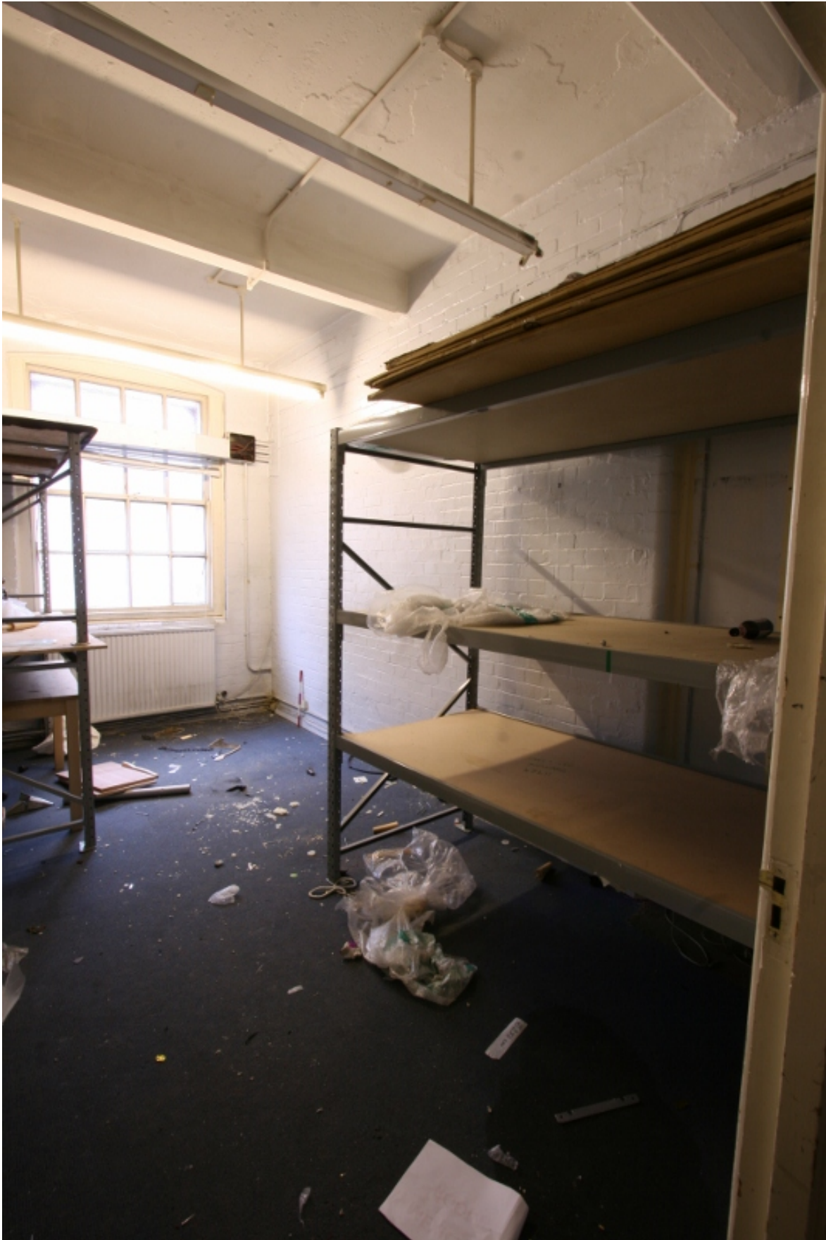
Plate 58: Ground floor room B2G12 with blocked doorway on right, looking north-west (VAL14 D100 (36))
