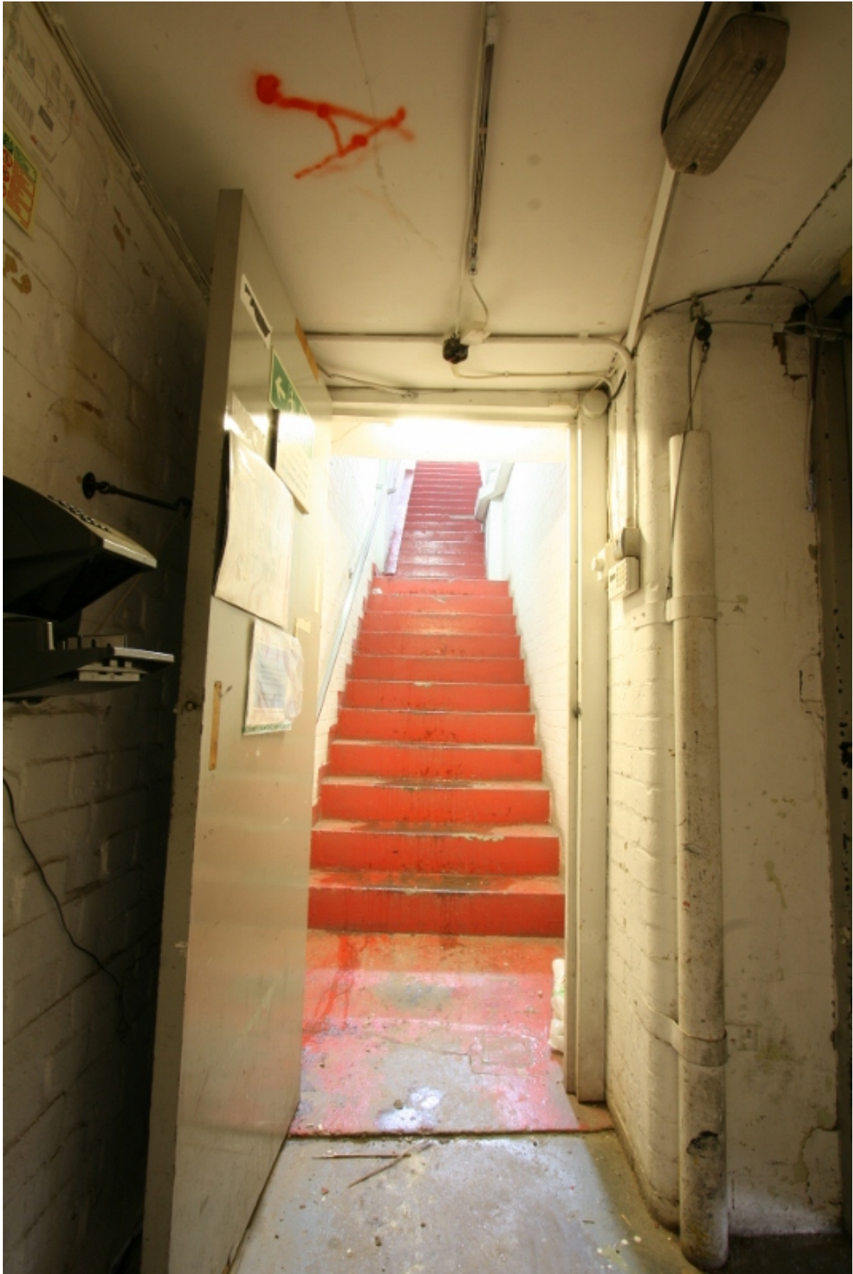
Plate 20: Stair access to first floor of nos 3-5 Valentine Place, looking west (VAL14 D100 (133))
