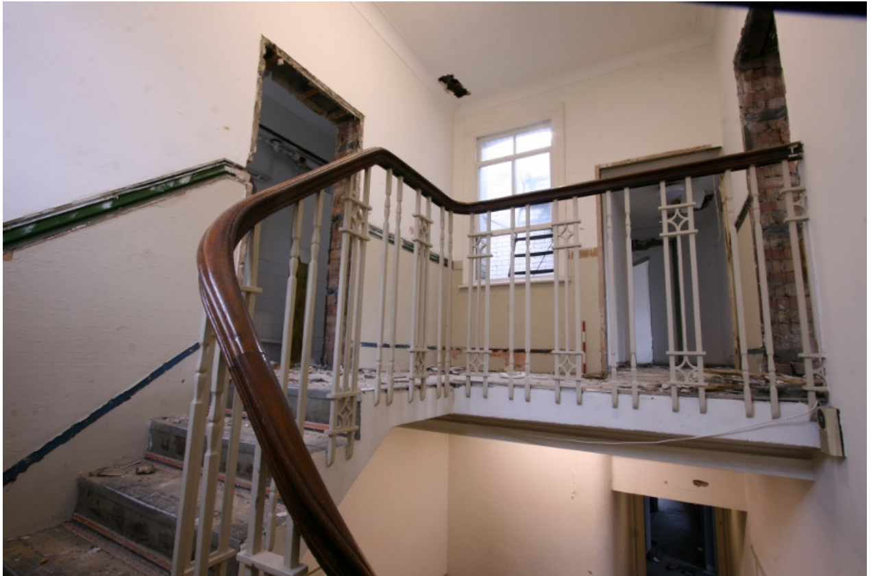
Plate 68: Original staircase (staircase 2) giving access from ground to first floor, looking north-east (VAL14 D100 (77))
