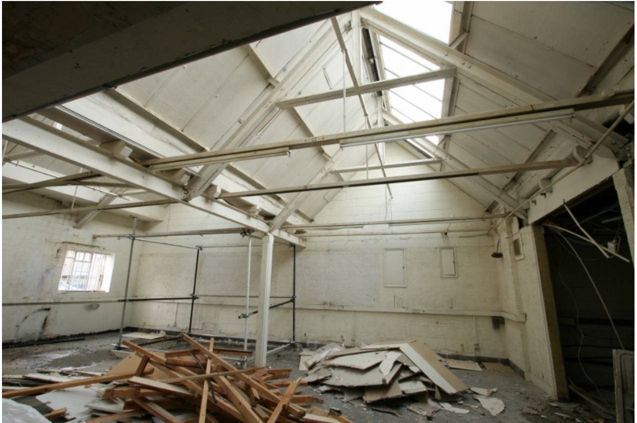
Plate 79: Exposed metal trusses of saw-tooth roof in room B2F10, looking south-east (VAL14 D100 (110))
