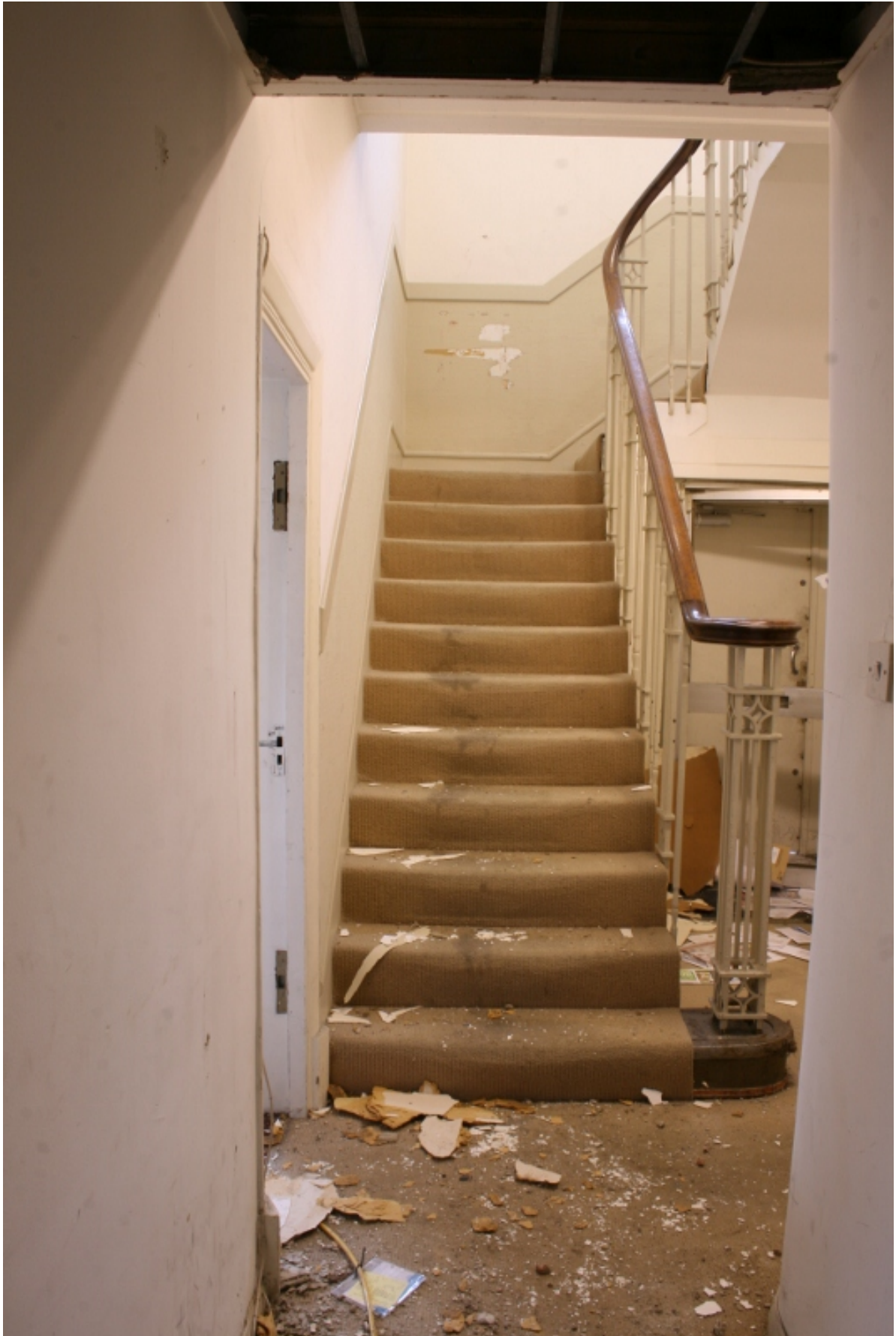
Plate 67: Original staircase (staircase 2) giving access from ground to first floor, looking west (VAL14 D100 (41))
