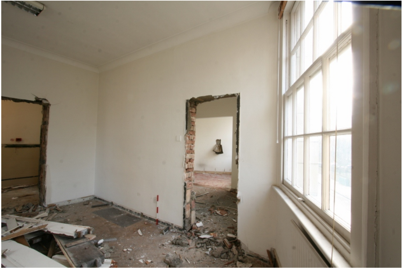
Plate 70: Removed fireplace indicated by original hearth stone in first floor room B2F4, looking north-east (VAL14 D100 (80))
