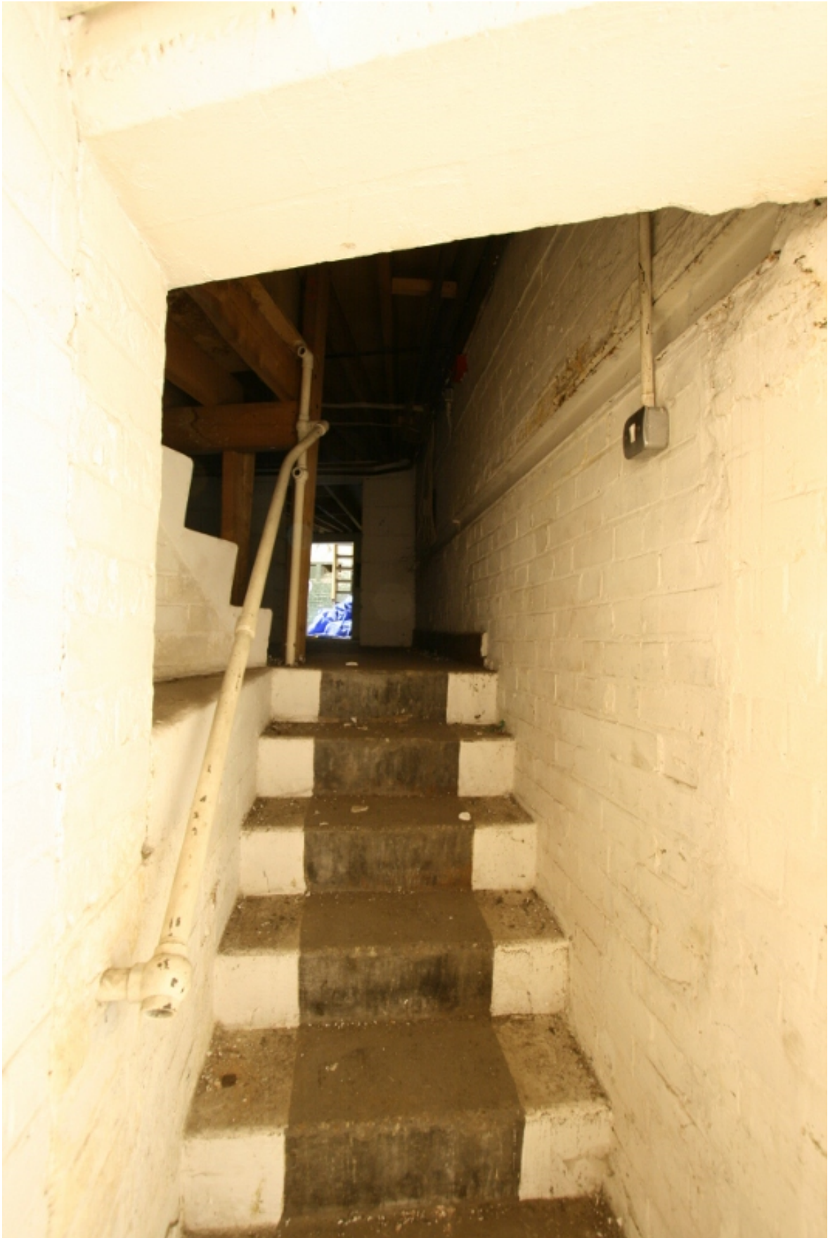
Plate 52: Disused stairwell leading from the basement to the ground floor, looking west (VAL14 D100 (62))
