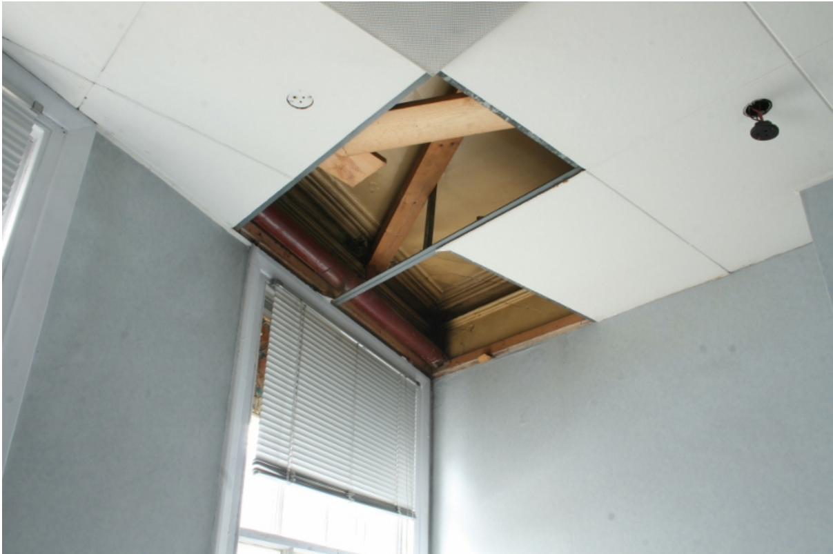
Plate 63: Exposed ceiling coving in ground floor room B2G17, looking south-west (VAL14 D100 (46))
