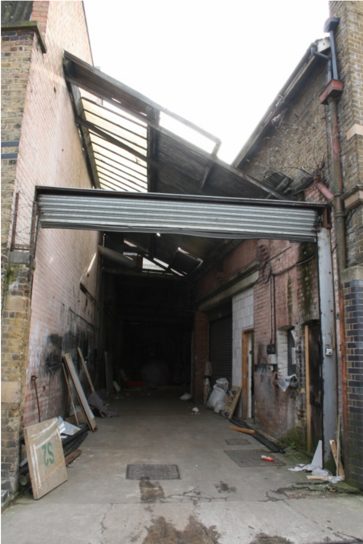
Plate 38: Covered access between nos 3-5 Valentine Place (left) and nos 17-19 Valentine Place/no. 21 Webber Street, looking west (VAL14 D100 (9))
