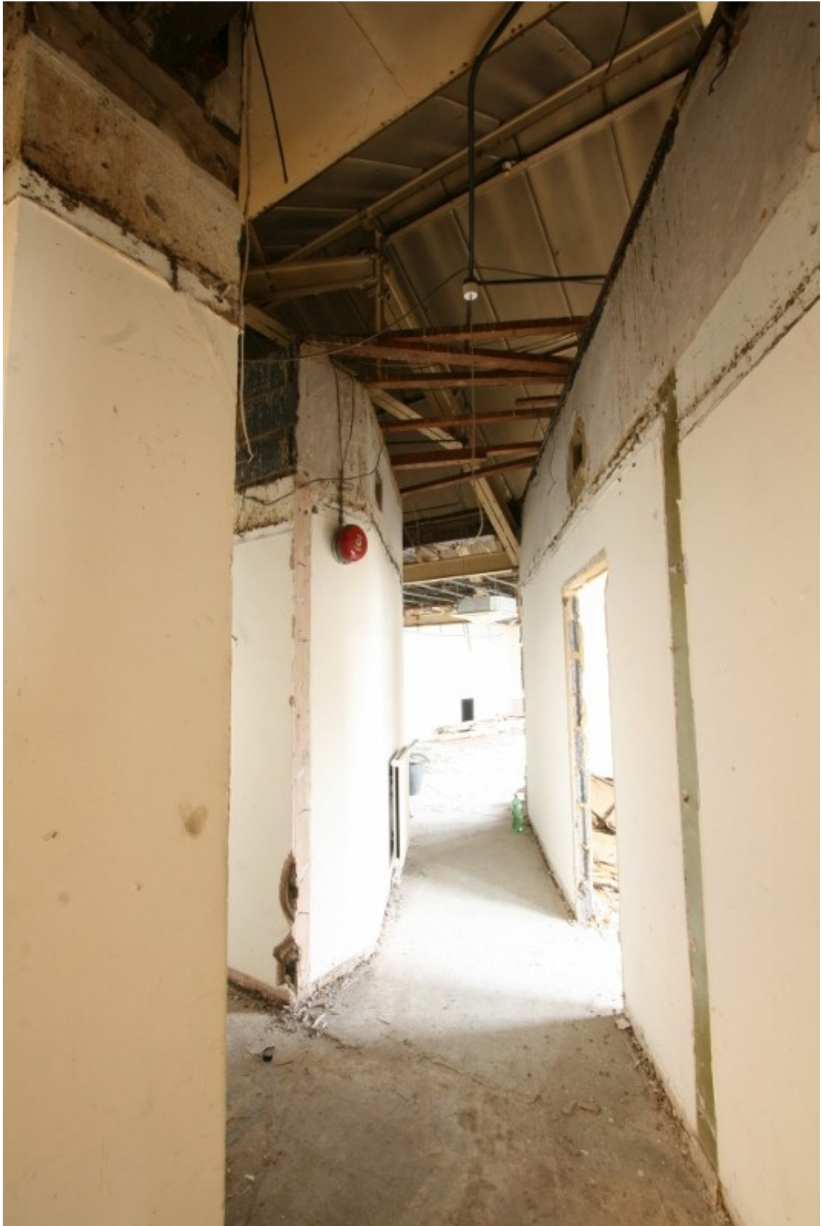
Plate 72: First floor corridor created by inserting modern partition concrete block walls, looking east (VAL14 D100 (118))
