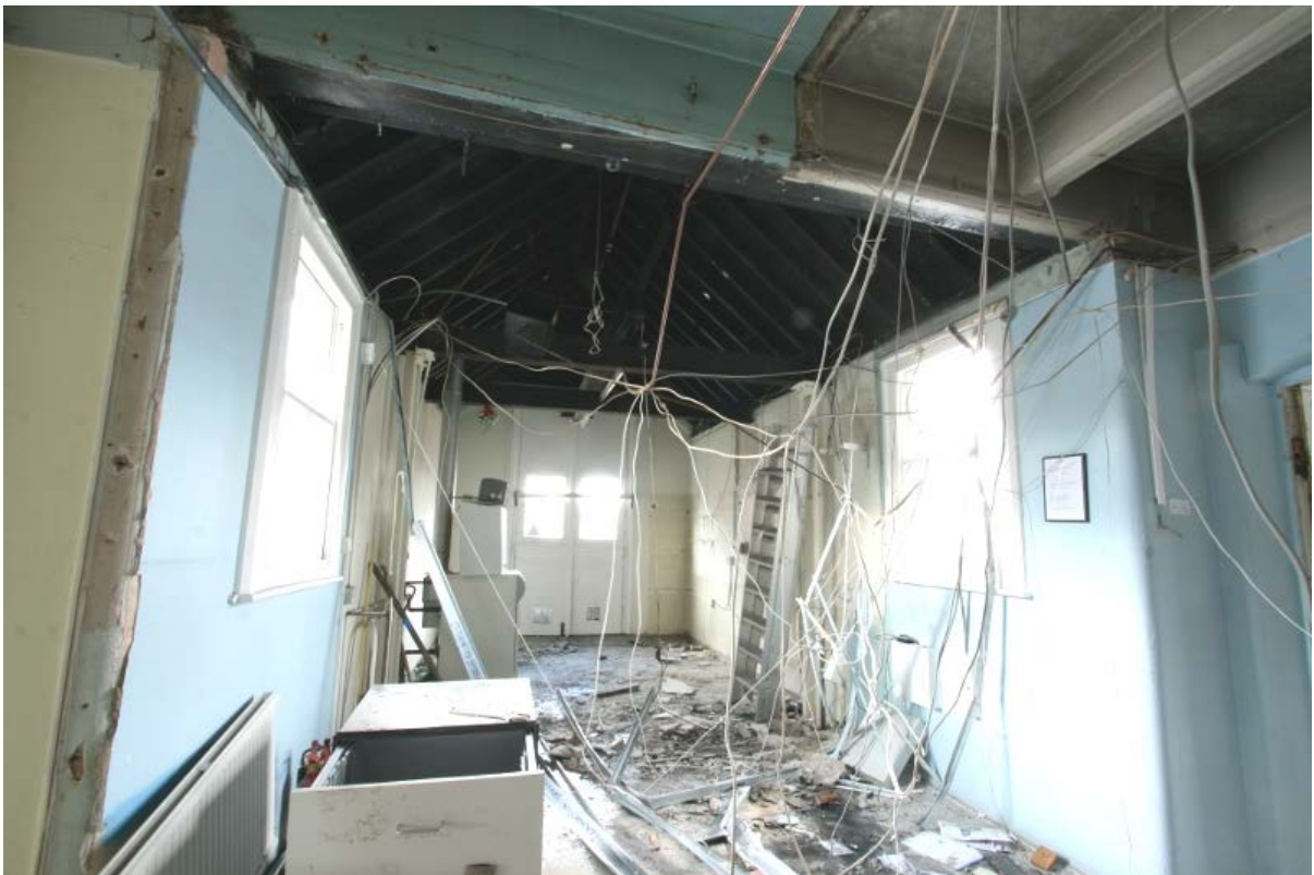
Plate 88: Original truss and part of winching gear in second floor room B2S3, looking west (VAL14 D100 (106))
