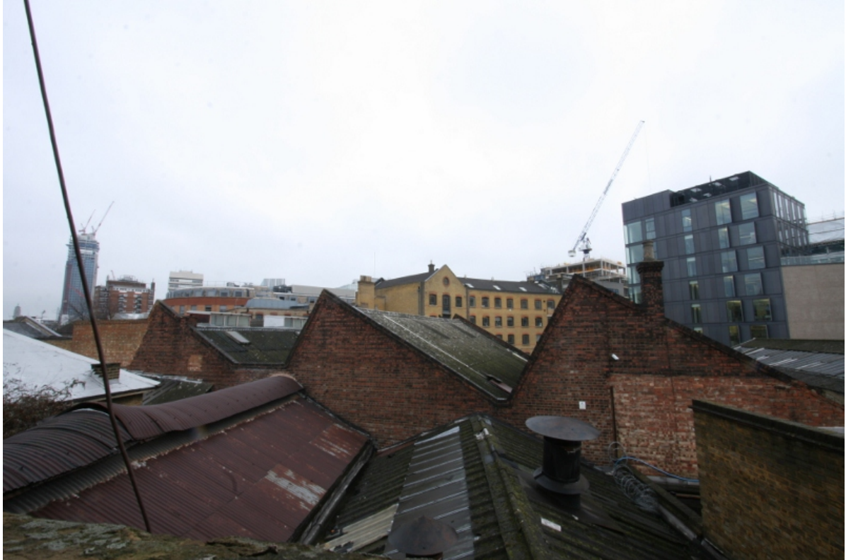
Plate 14: South elevation of nos 3-5 Valentine Place showing saw-tooth roof, looking north (VAL14 D100 (122))
