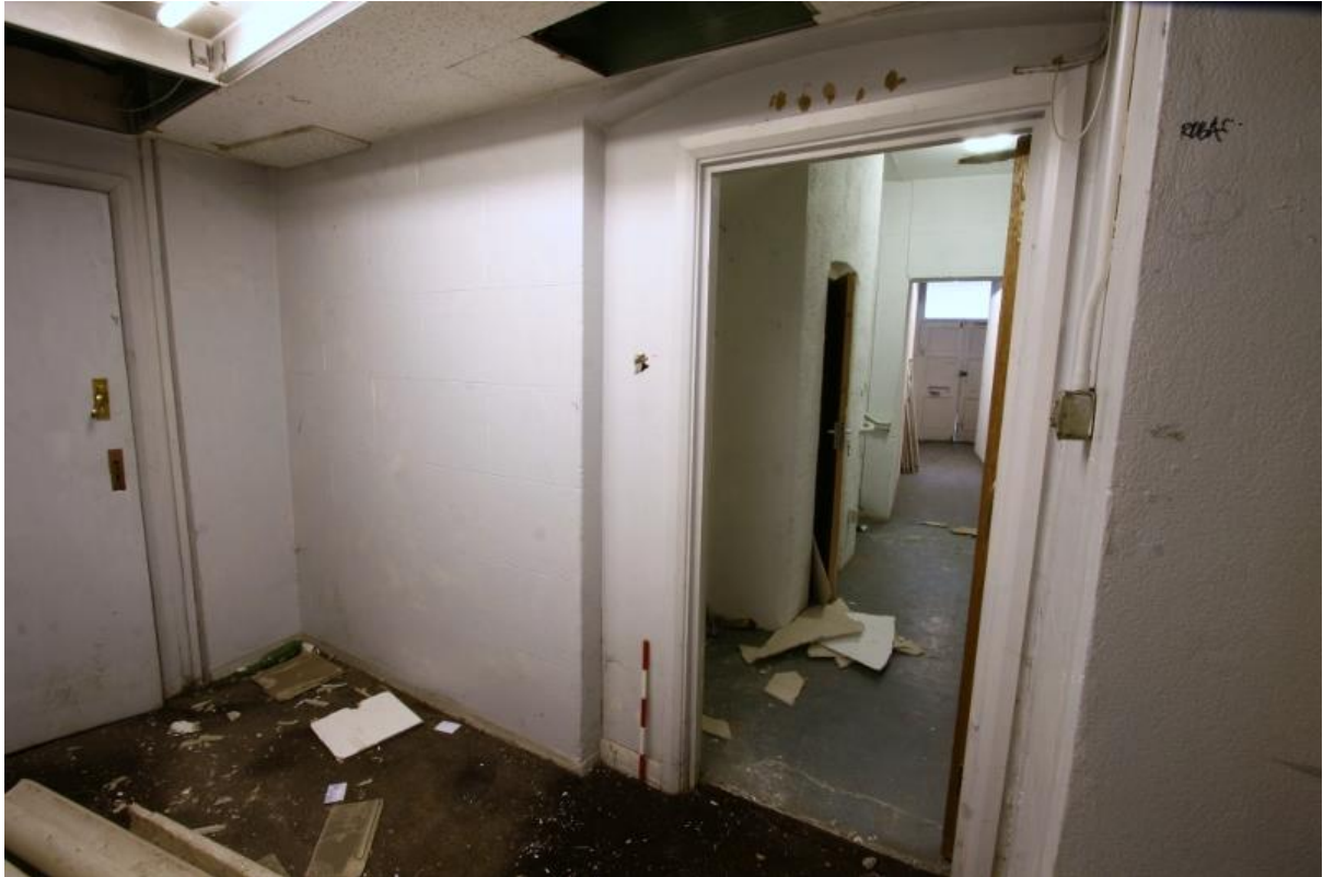
Plate 53: Northern end of ground floor corridor 2 adjacent to stairwell 1, looking east (VAL14 D100 (28))
