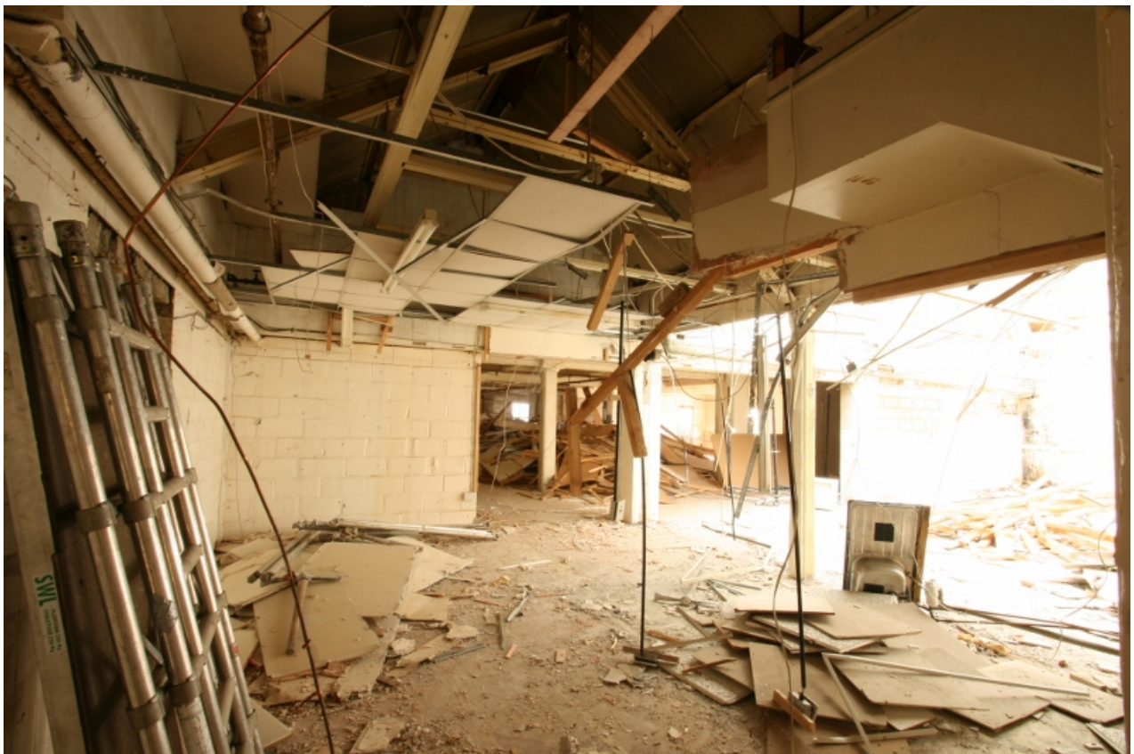
Plate 80: Exposed roof truss structure in first floor room B2F9 following partial soft strip, looking north-east (VAL14 D100 (107))
