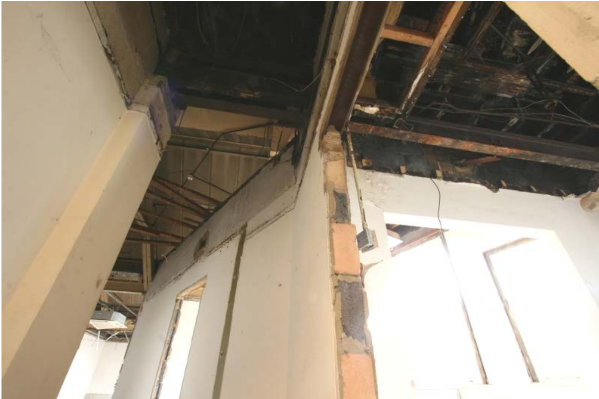
Plate 73: Exposed metal roof trusses and ceiling timbers in first floor rooms B2F7 and B2F8, looking east (VAL14 D100 (119))
