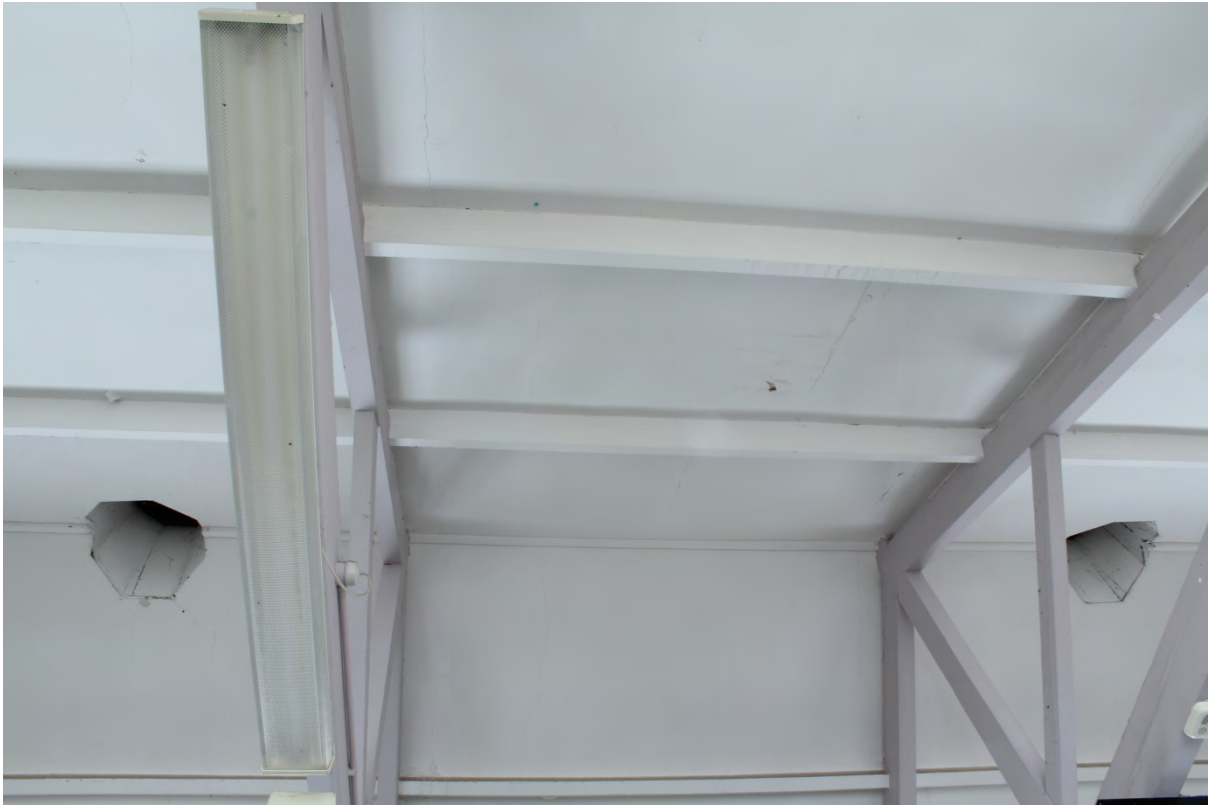
Plate 26: Ceiling vents, looking up and west (WDS15 D1 (41))
