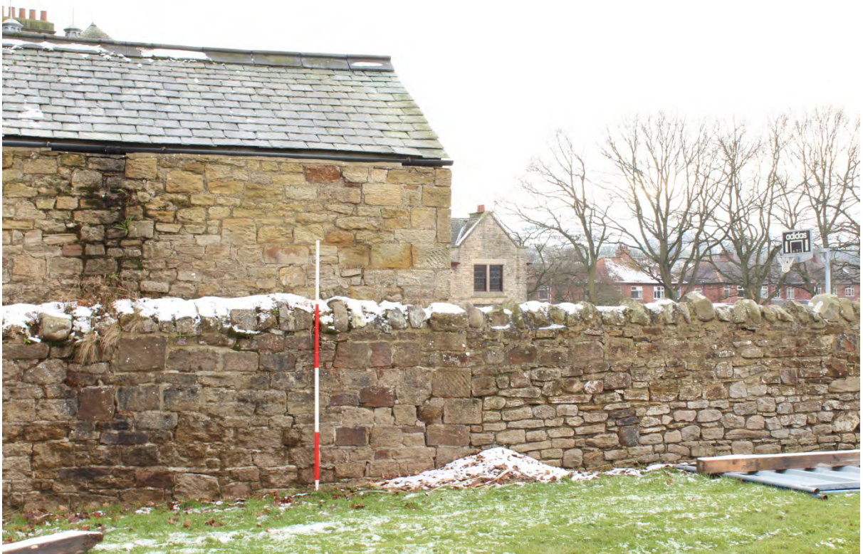
Plate 9: Detail of low perimeter wall showing change in stone size, looking south-west (WDS15 D1 (30))
