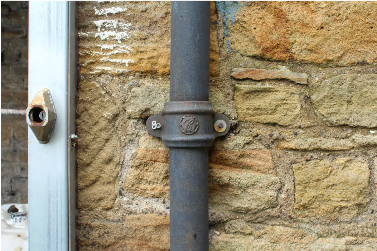
Plate 38: Detail of iron downpipe on exterior of converted outbuilding, looking north (WDS15 D1 (25))
